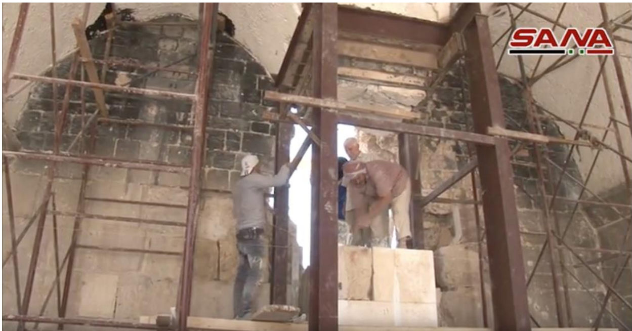
A video still of workers replacing stones at the al-Umayyad Mosque (SANA; September 25, 2018)
