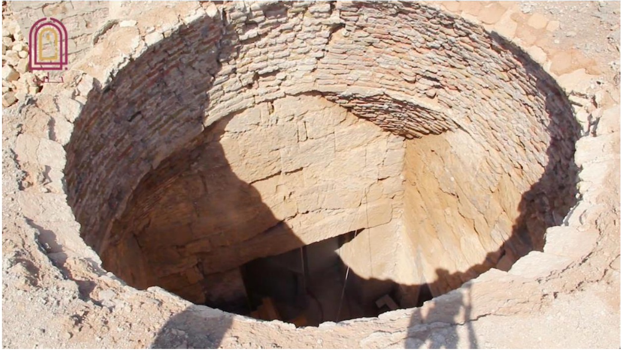
A video still of a missing dome at the al-Kabir Mosque (Bawaba Halab; September 6, 2018)
