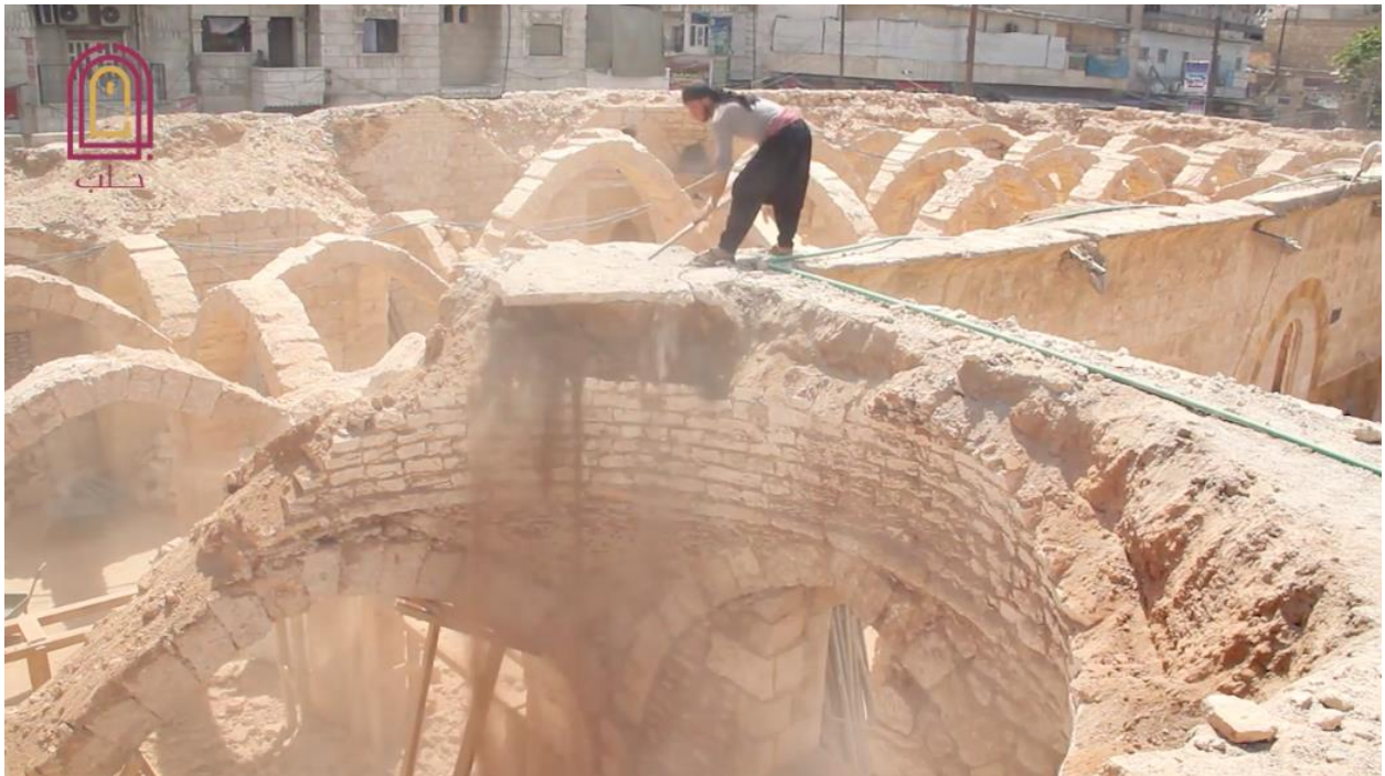
Video still of a worker removing damaged architecture at the al-Kabir Mosque (Bawaba Halab; September 6, 2018)
