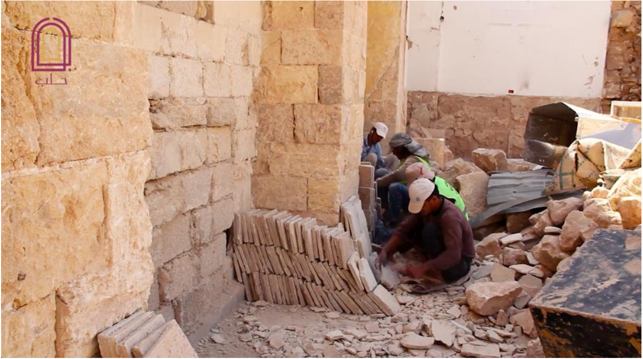
Video still of workers cleaning and stacking tiles at the al-Kabir Mosque (Bawaba Halab; September 6, 2018)
