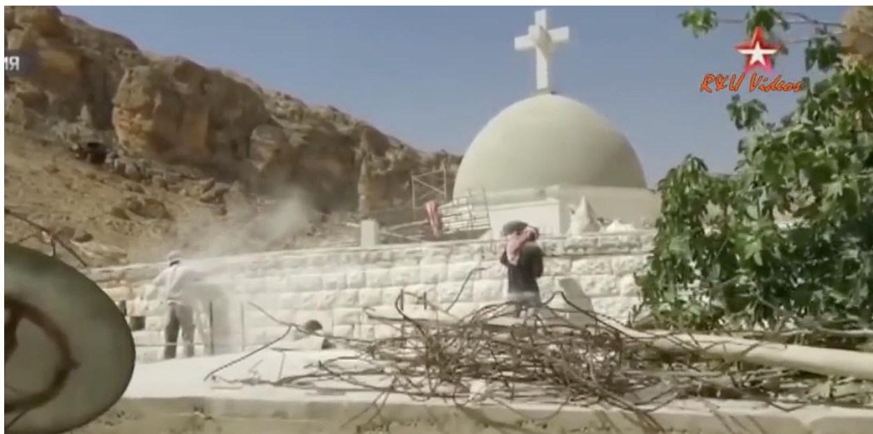
A video still of repair work at the St. George Church (R&U Videos; September 6, 2018)
