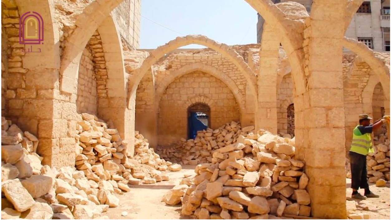
Video still of workers and organized stones at the al-Kabir Mosque (Bawaba Halab; September 6, 2018)
