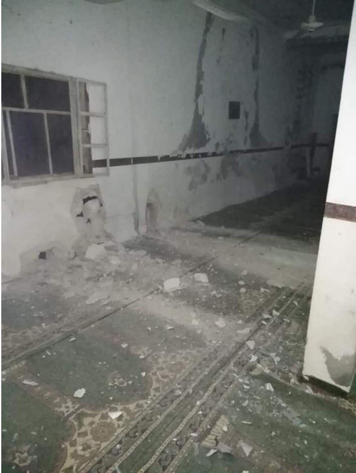
Damage to a wall in the mosque (Media Center in Talafah Village; November 20, 2018)
