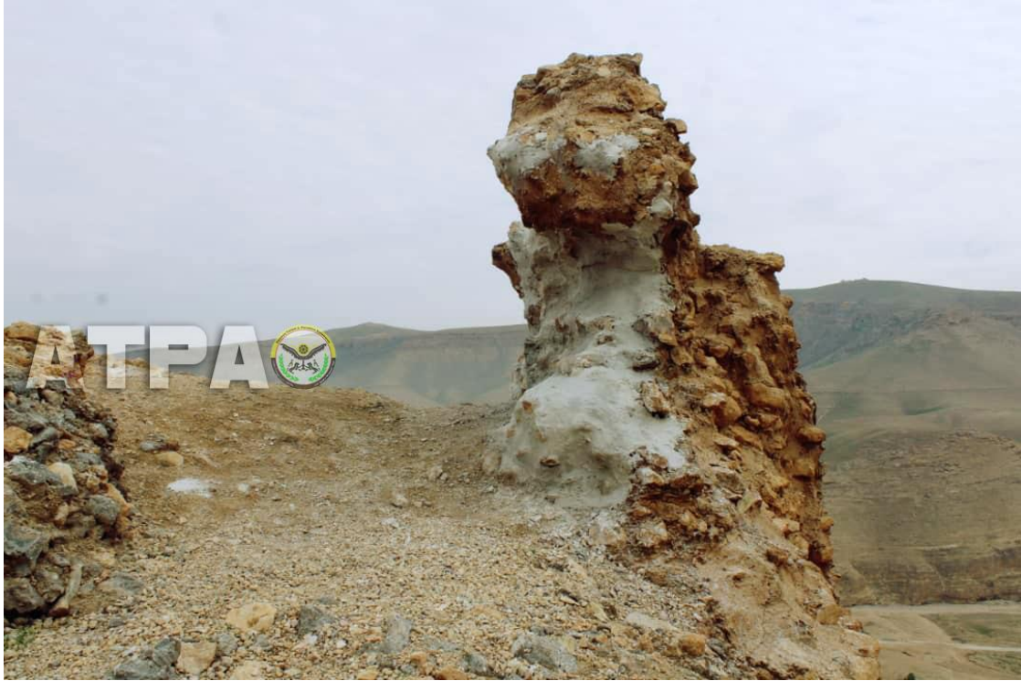
Conservation work at Qalaat Sukara with the application of plaster to stabilize the bricks (ATPA; November 26, 2018)
