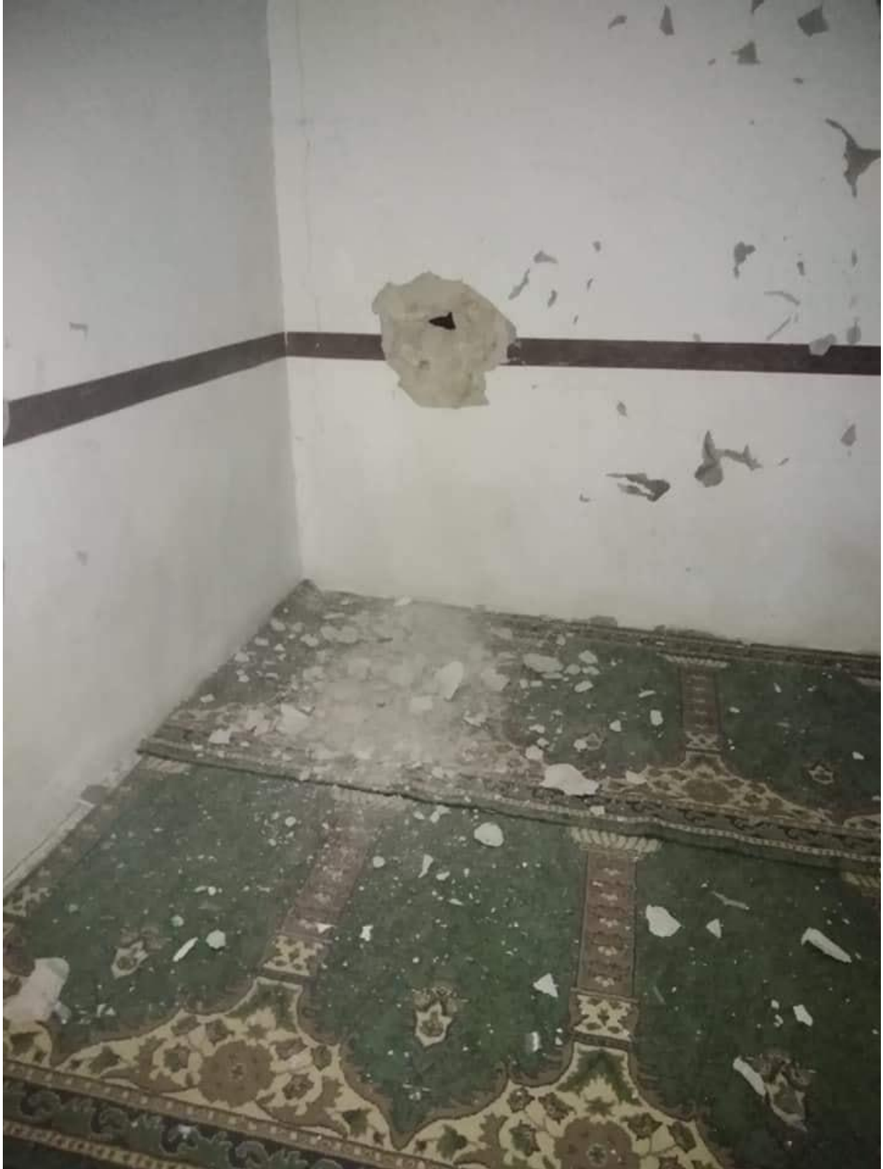
Damage to a wall in the mosque (Media Center in Talafah Village; November 20, 2018)
