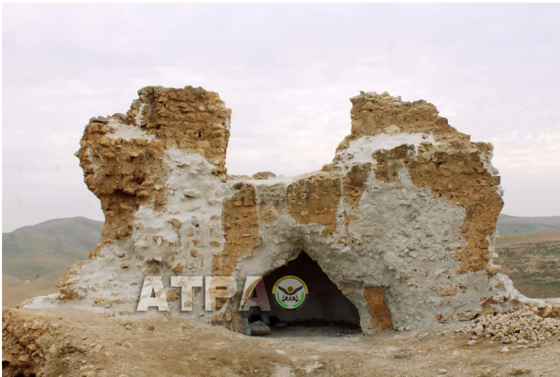
Conservation work at Qalaat Sukara with the application of plaster to stabilize the bricks (ATPA; November 26, 2018)
