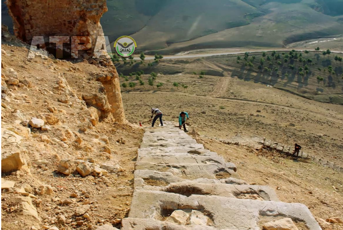
The cleaning of the steps leading up to Qalaat Sukara (ATPA; November 15, 2018)
