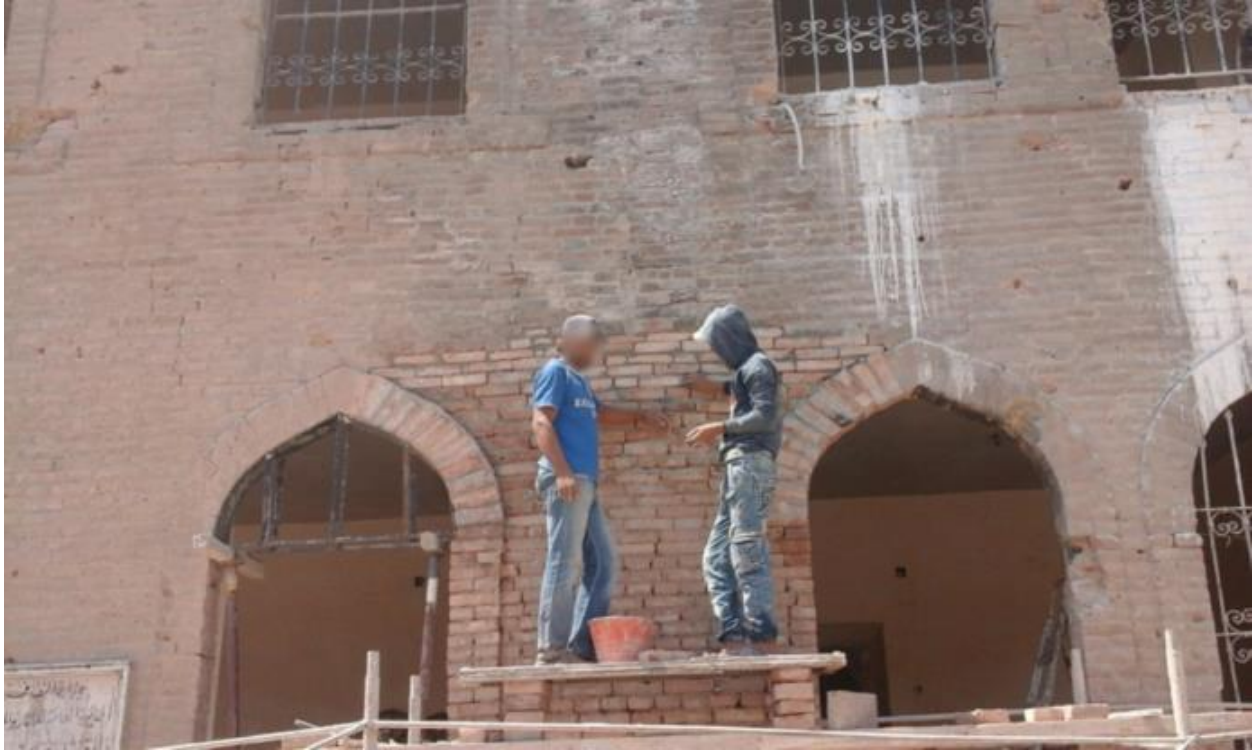
The repaired east wall of the Raqqa Museum using bricks from the refurbished Heraqla Brickyard (ASOR CHI).
