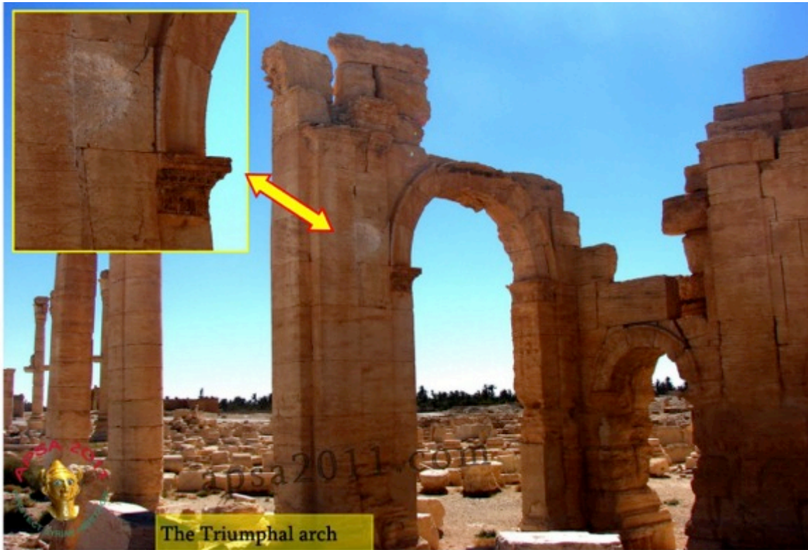
Figure 49: Shell damage to facade of the small northeastern arch next to the triumphal arch (Source: APSA)
