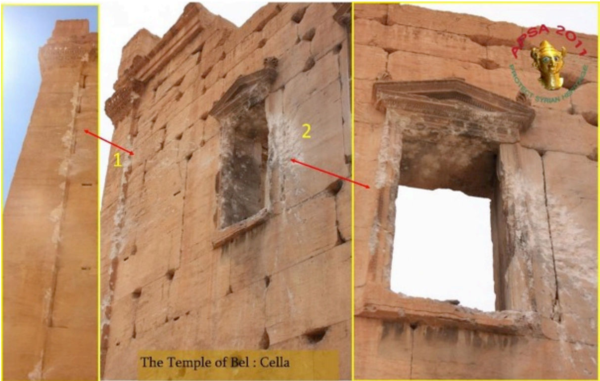
Figure 42: Sanctuary of the temple, damage to the southeastern corner of the eastern wall (Source: APSA)
