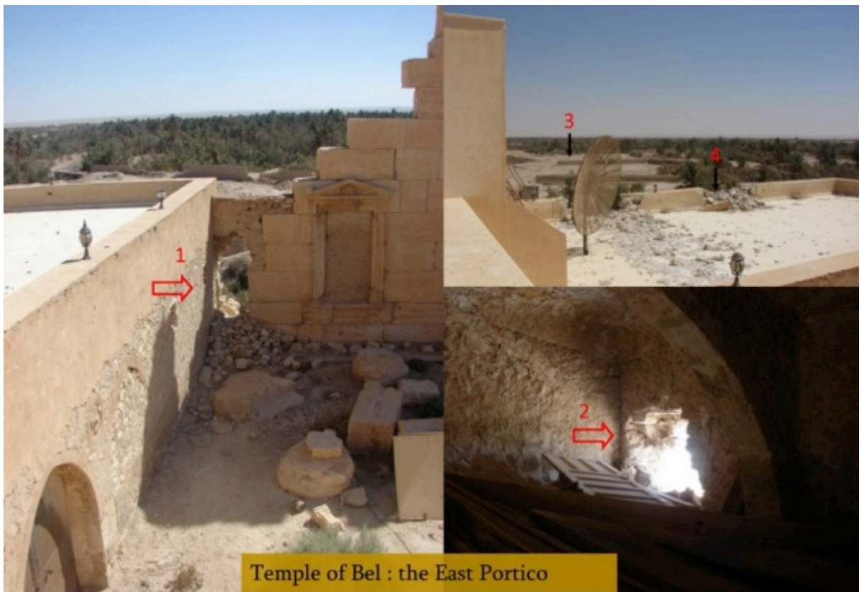
Figure 35: The two openings created by thieves at the southeastern corner of the enclosure of the temple of Baal (Source: APSA)
