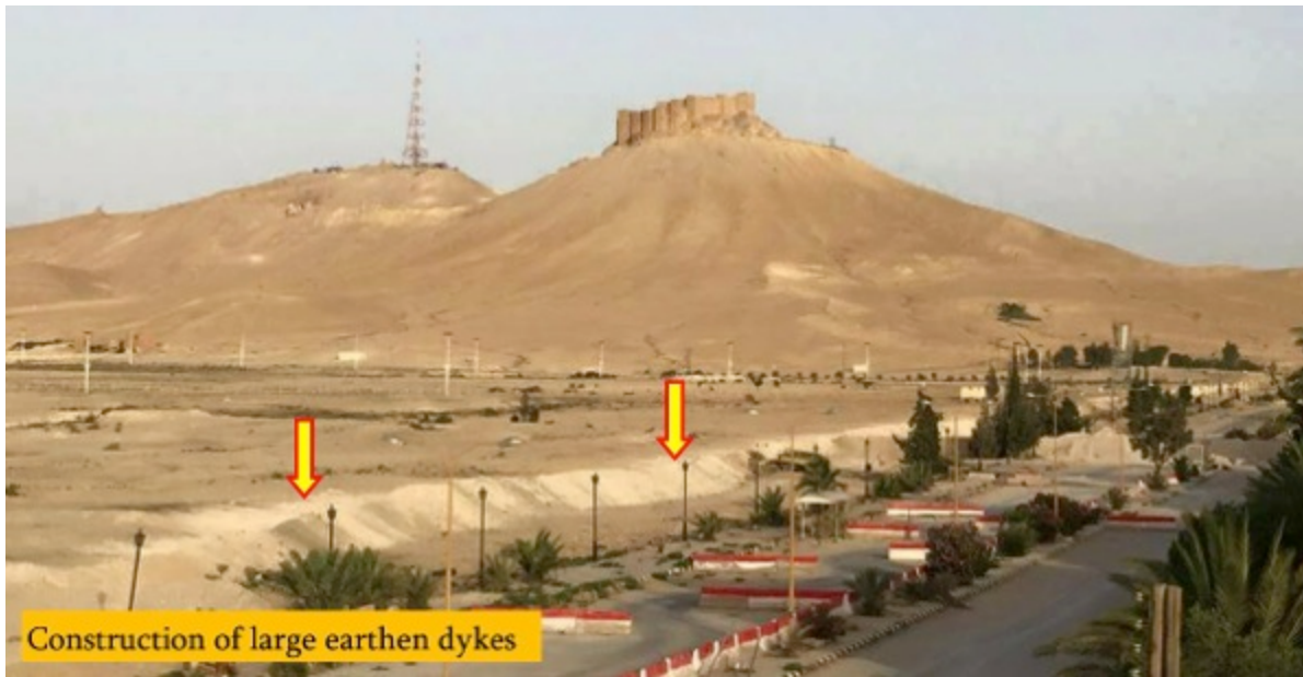
Figure 8: Levee in the archaeological area near the police station (Source: Coordination of the City of Palmyra)
