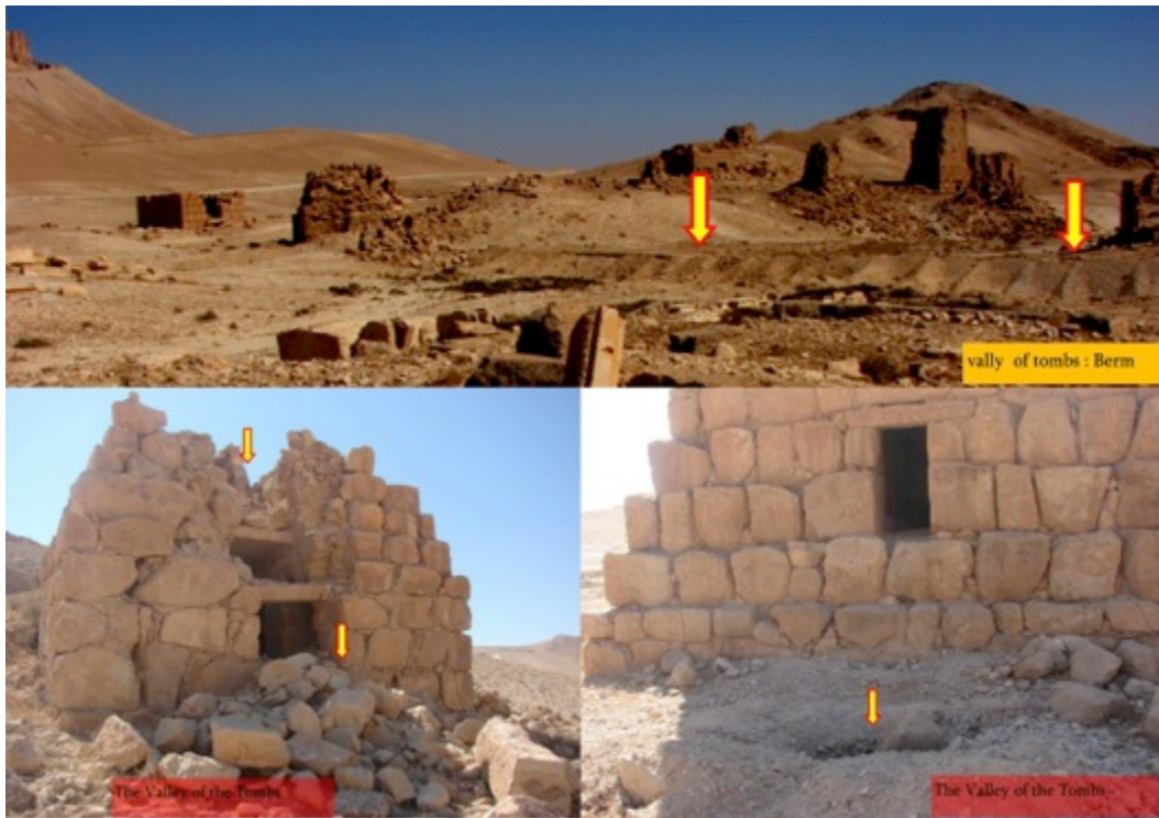
Figure 59: Some damage in the area of Valley of the Tombs area (Source: APSA)
