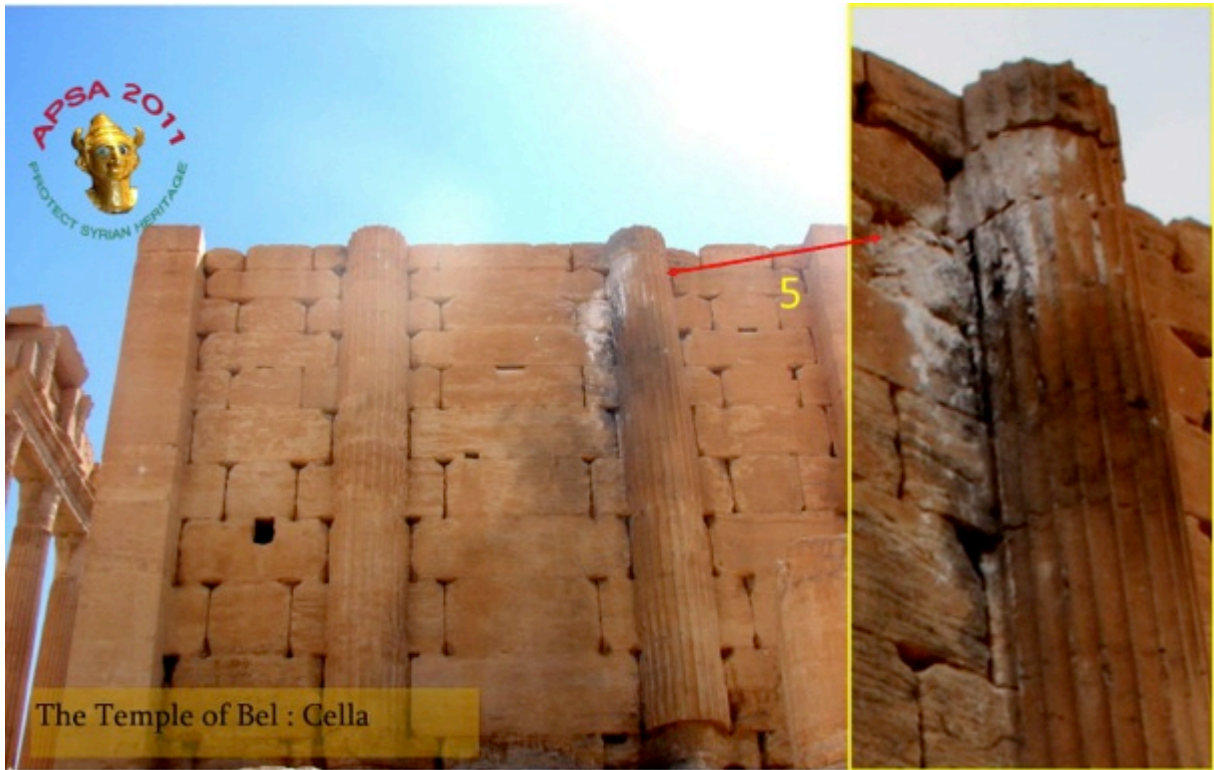
Figure 47: Sanctuary of the temple, crumbling of the upper part of a column and the northern wall, Point no. 5 (Source: APSA)
