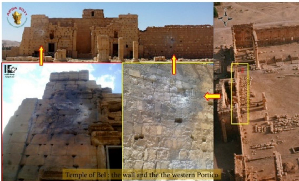
Figure 20: Damage to the interior facade of the western wall (Source: APSA and Lens Young Tadmouri)
