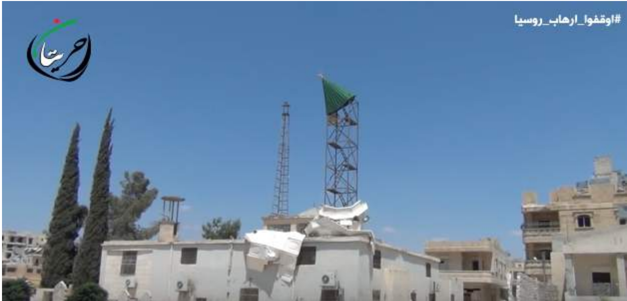
Video still of damage to Ali Sayyad Mosque and minaret (Hraytan City; June 30, 2016)
