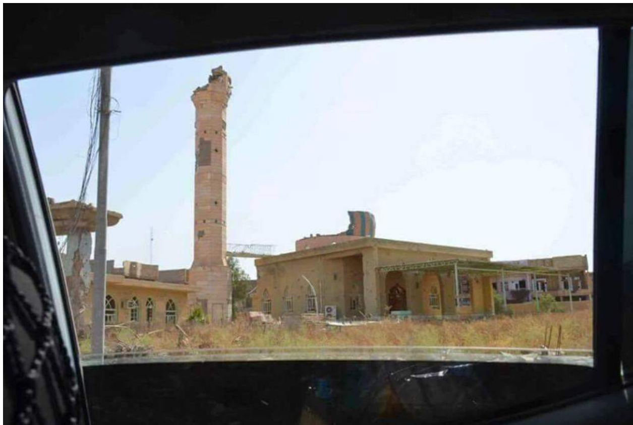
Severe damage to minaret and dome of al-Hassan al-Basri Mosque (Twitter; June 23, 2016)
