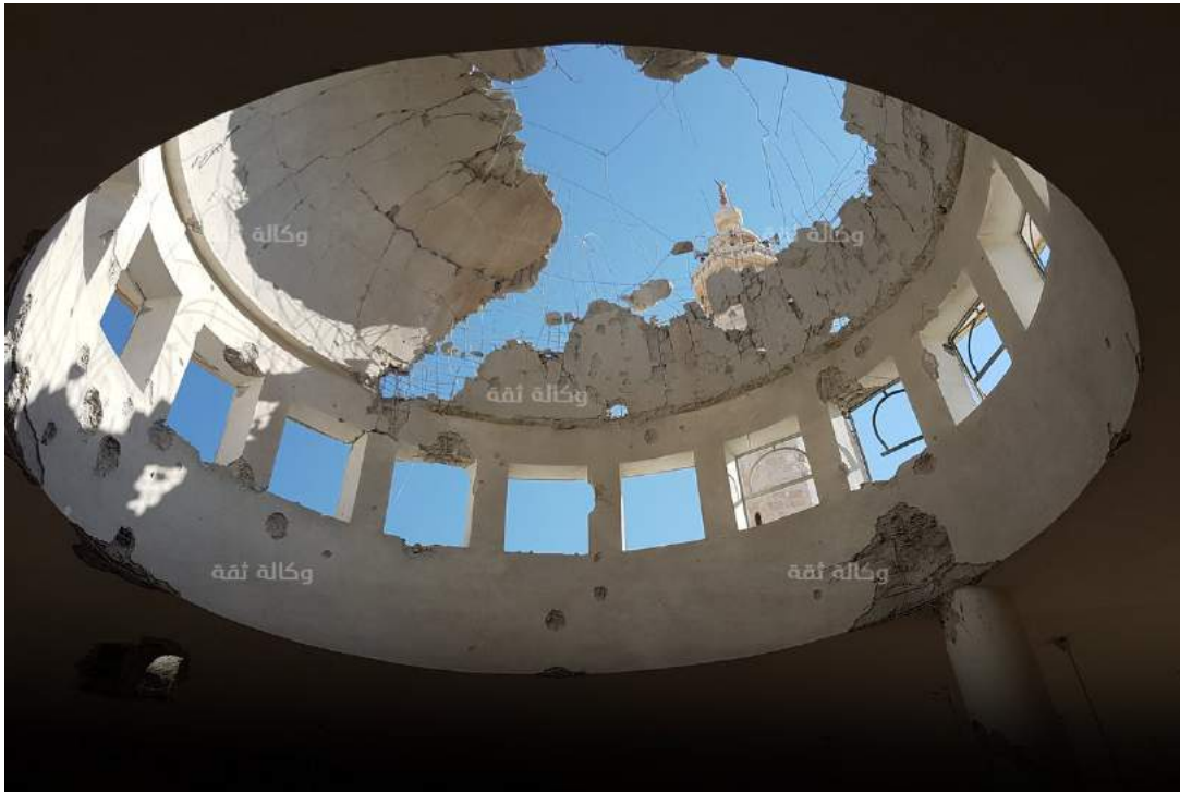
Damage to the interior of the dome of al-Farouq Mosque (Thiqa News Agency; July 1, 2016)
