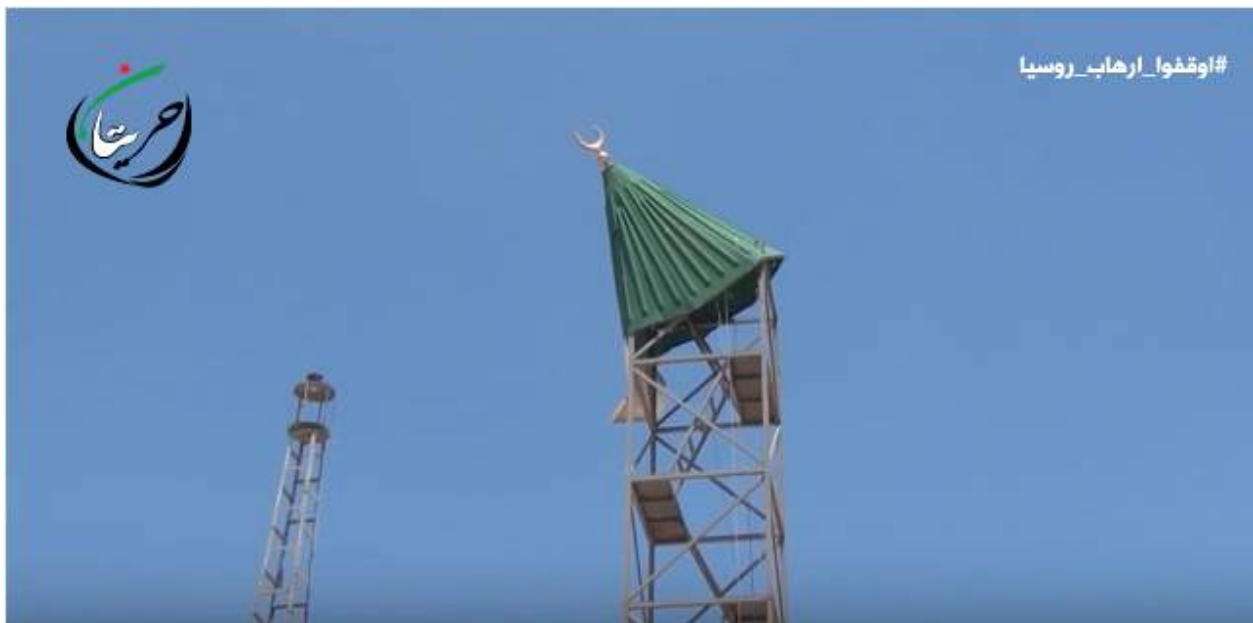
Detail of damage to the minaret, the facade of which has fallen off its metal supports (Hraytan City; June 30, 2016)
