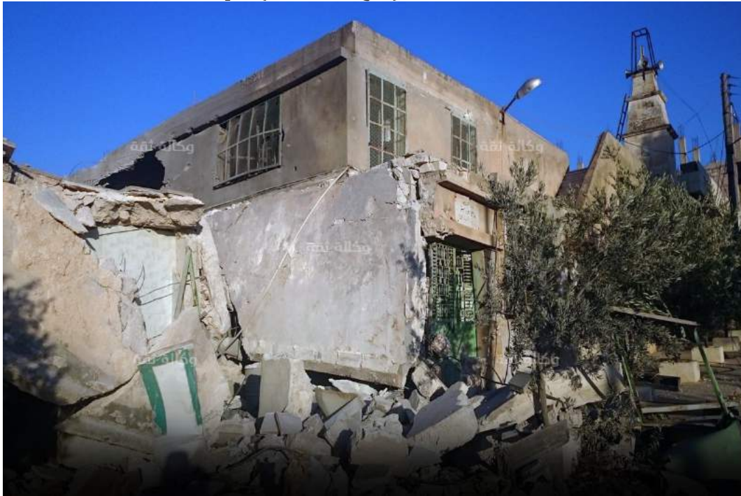
Exterior view of damage to Ammar bin Yasser Mosque (Thiqa News Agency; July 1, 2016)
