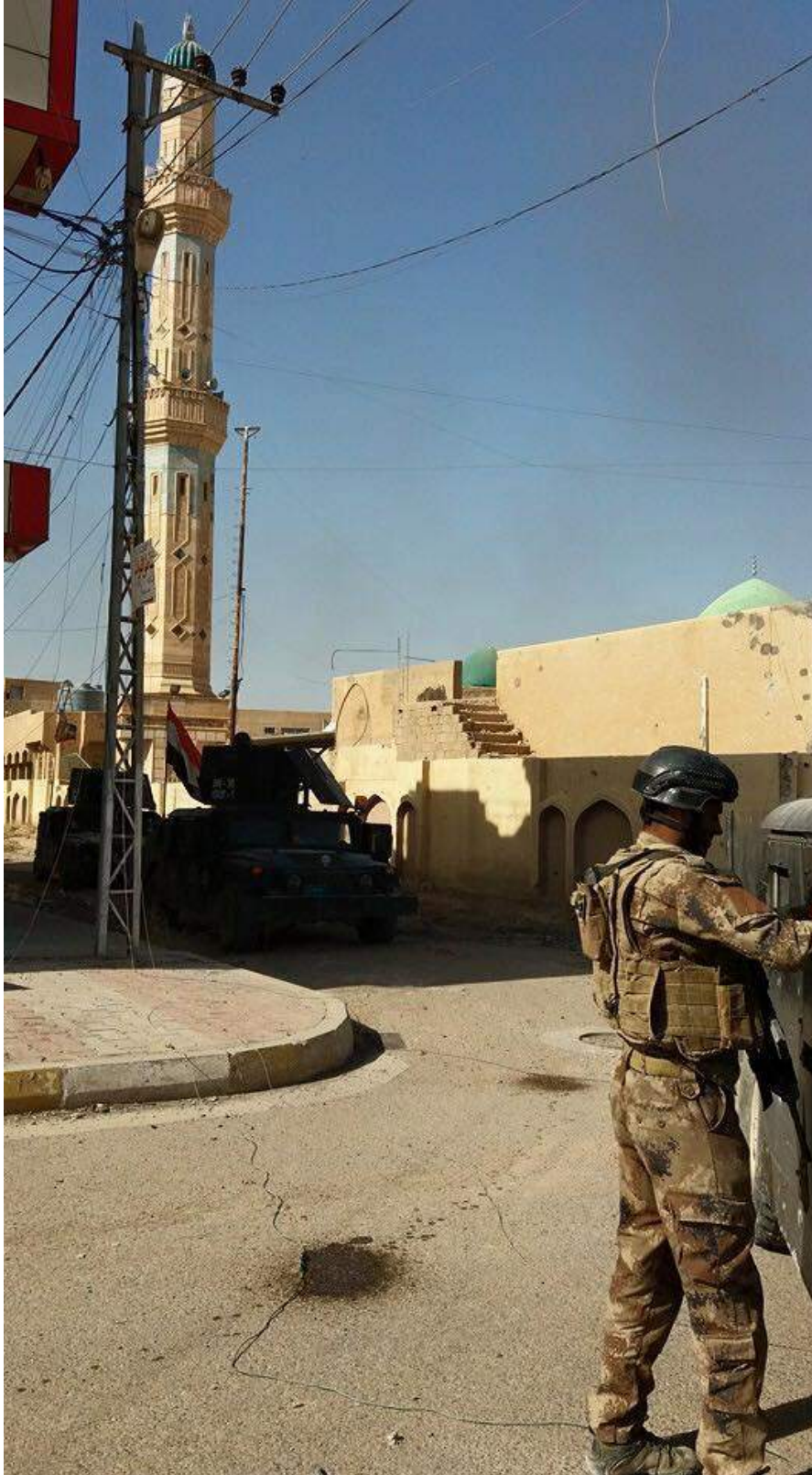
Minor exterior damage to al-Sheikh Abdul Aziz al-Samarrai Mosque (Iraqi PMU English; June 18, 2016)
