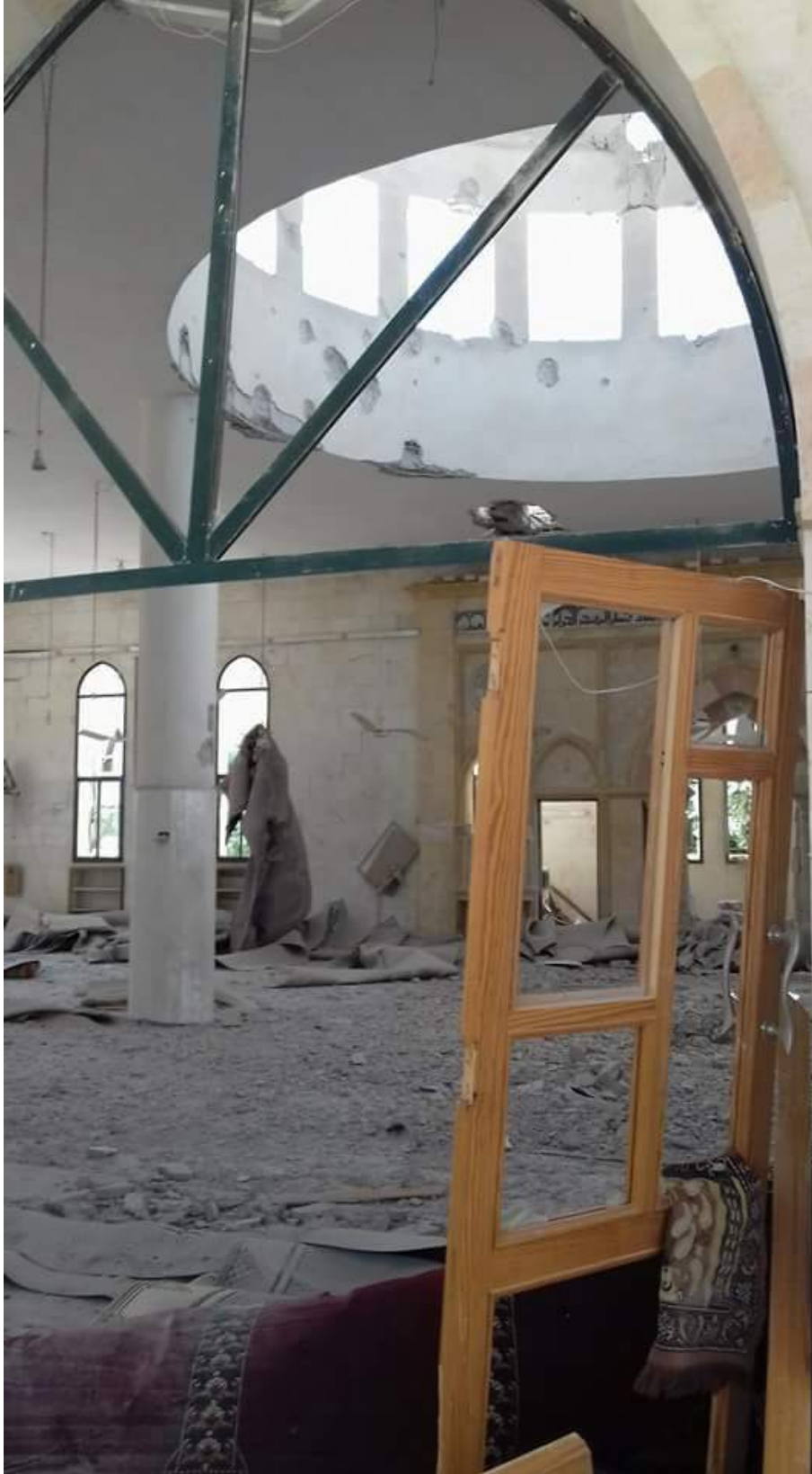
Interior and material damage to al-Farouq Mosque (Kafr Hamra Media Center; June 30, 2016)
