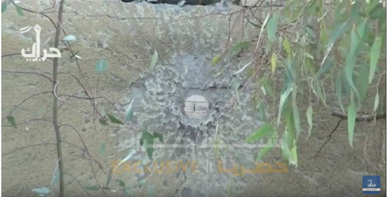
Damage to al-Hassan al-Basri Mosque complex wall (Herak News; February 20, 2014)
