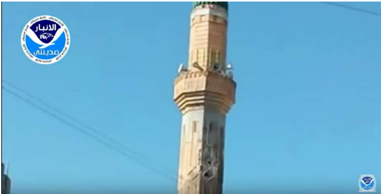
Minor damage to minaret of al-Sheikh Abdul Aziz al-Samarrai Mosque (Anbar Cities; October 17, 2014)
