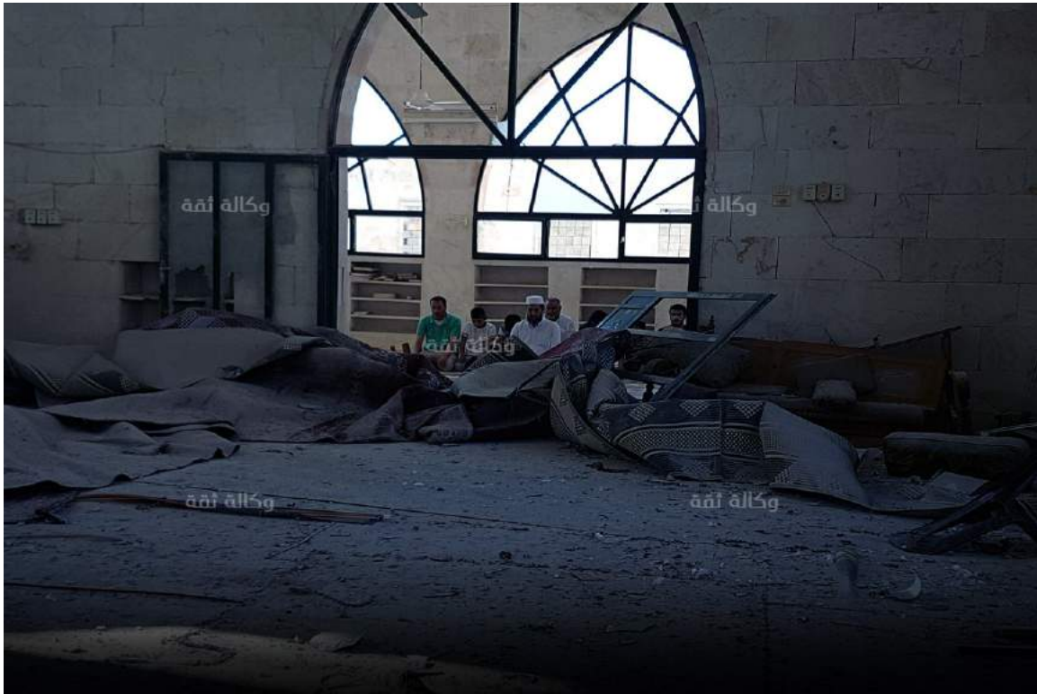
Damage to the interior of al-Farouq Mosque (Thiqa News Agency; July 1, 2016)
