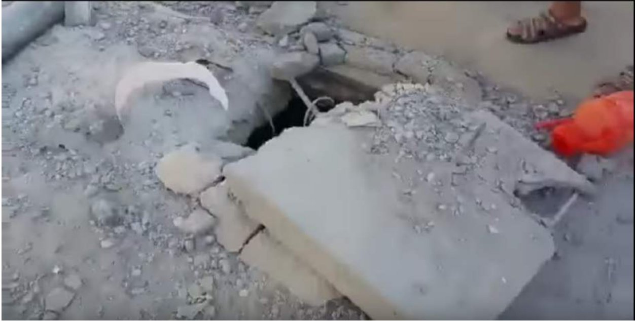
Damage to the exterior of the courtyard of Abu Obeida Mosque (Iraqi Spring Media Center; May 21, 2016)
