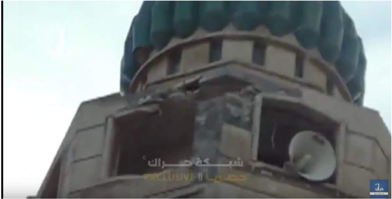
Damage to al-Hassan al-Basri Mosque minaret (Herak News; January 14, 2014)
