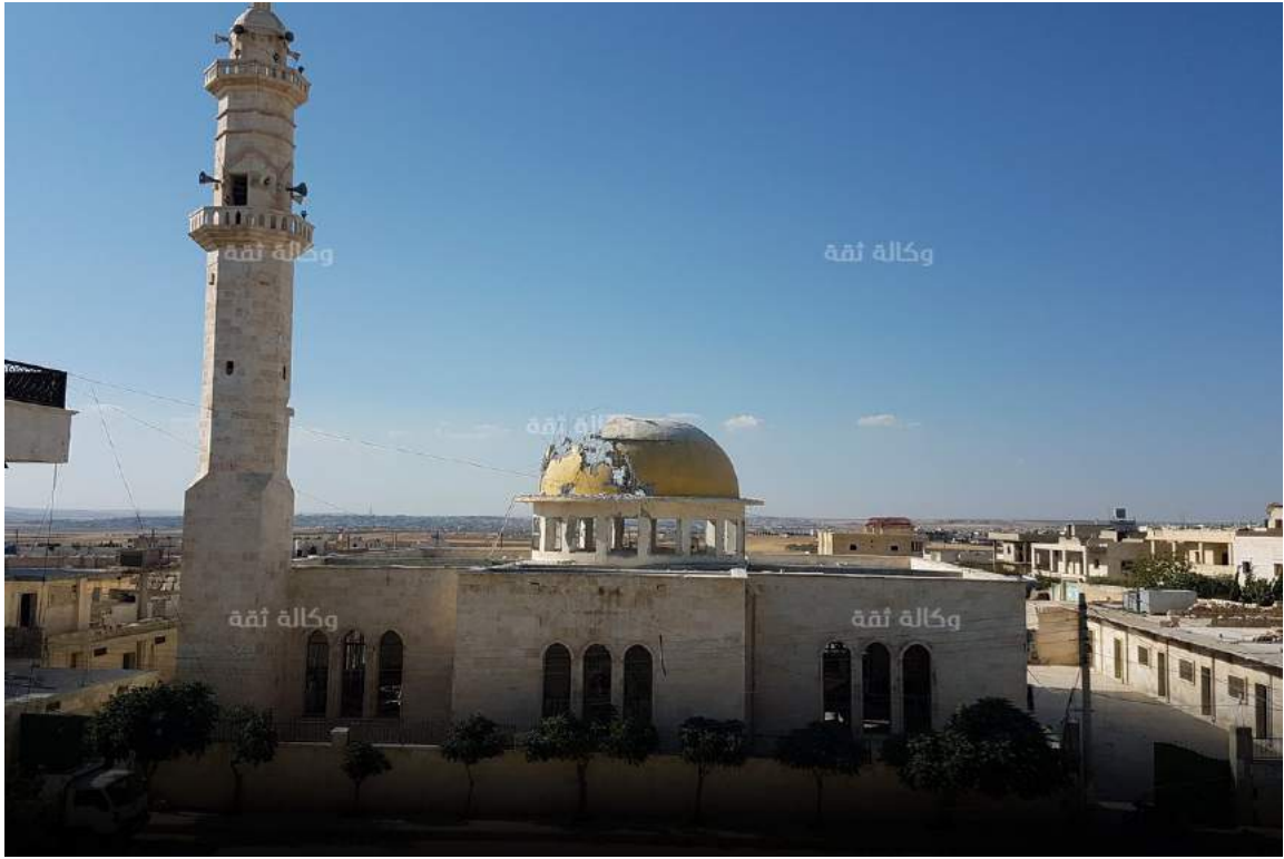
Damage to al-Farouq Mosque (Thiqa News Agency; July 1, 2016)
