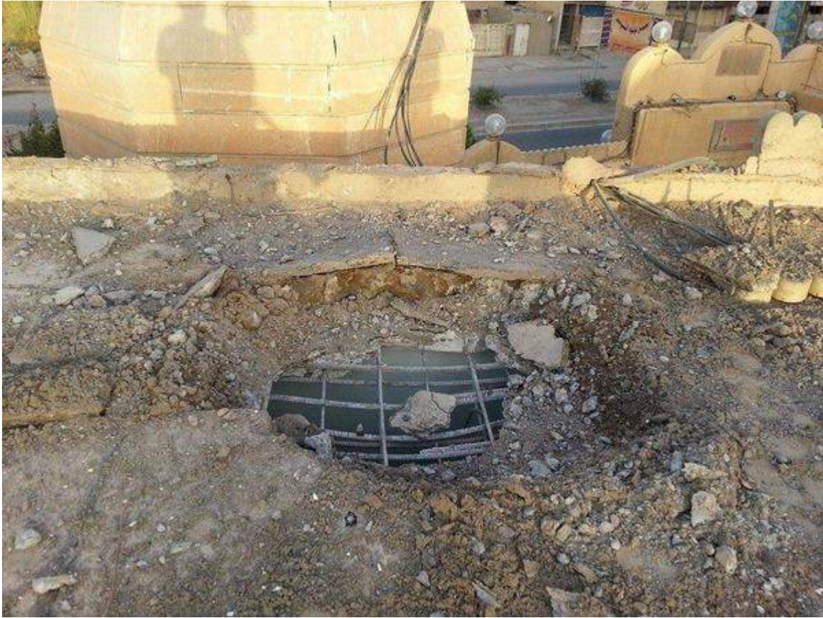
A hole in the roof of al-Furqan Mosque following an airstrike (Twitter; September 23, 2014)
