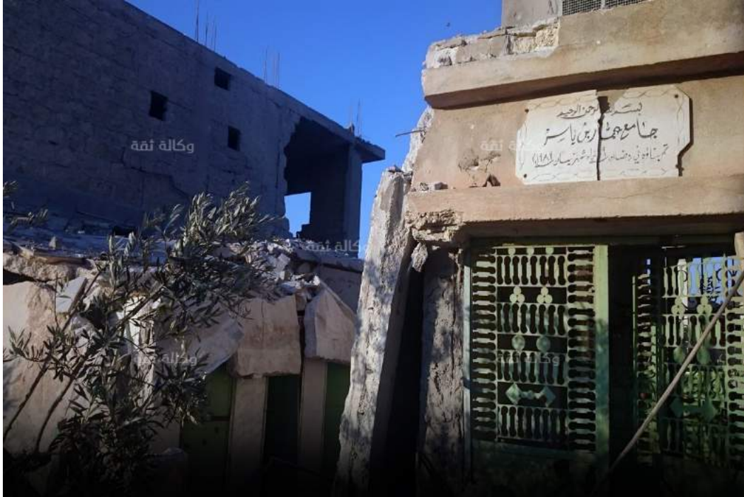
Exterior view of damage to Ammar bin Yasser Mosque (Thiqa News Agency; July 1, 2016)
