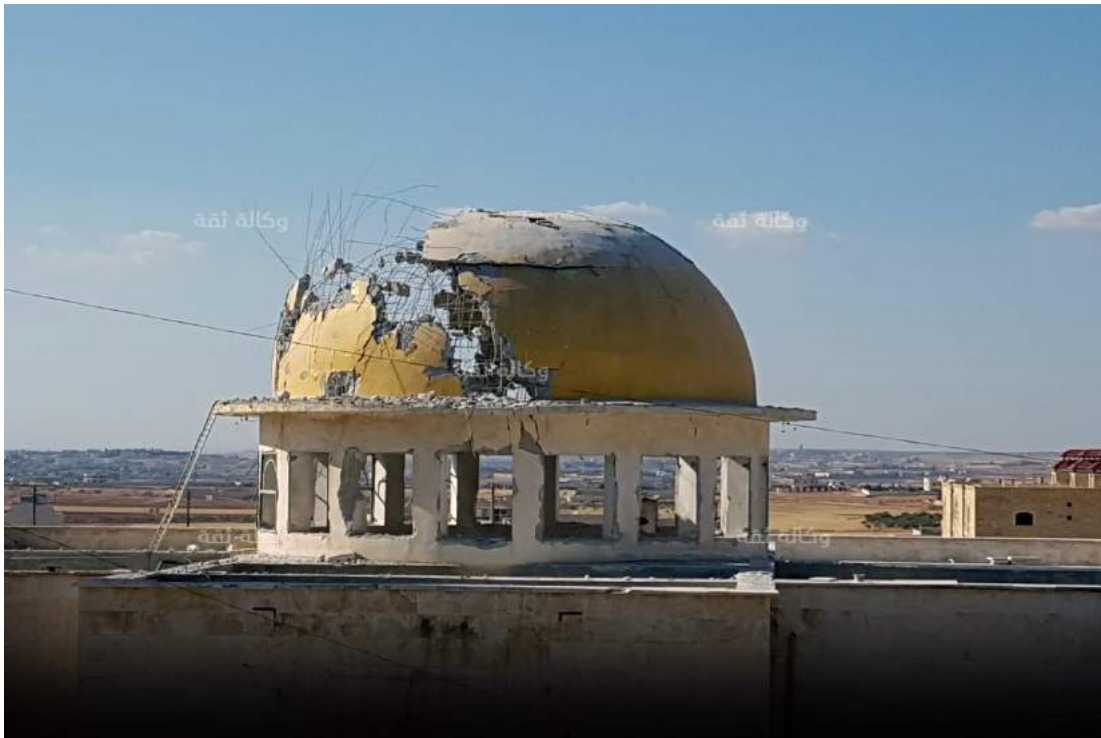
Damage to the exterior of the dome of al-Farouq Mosque (Thiqa News Agency; July 1, 2016)
