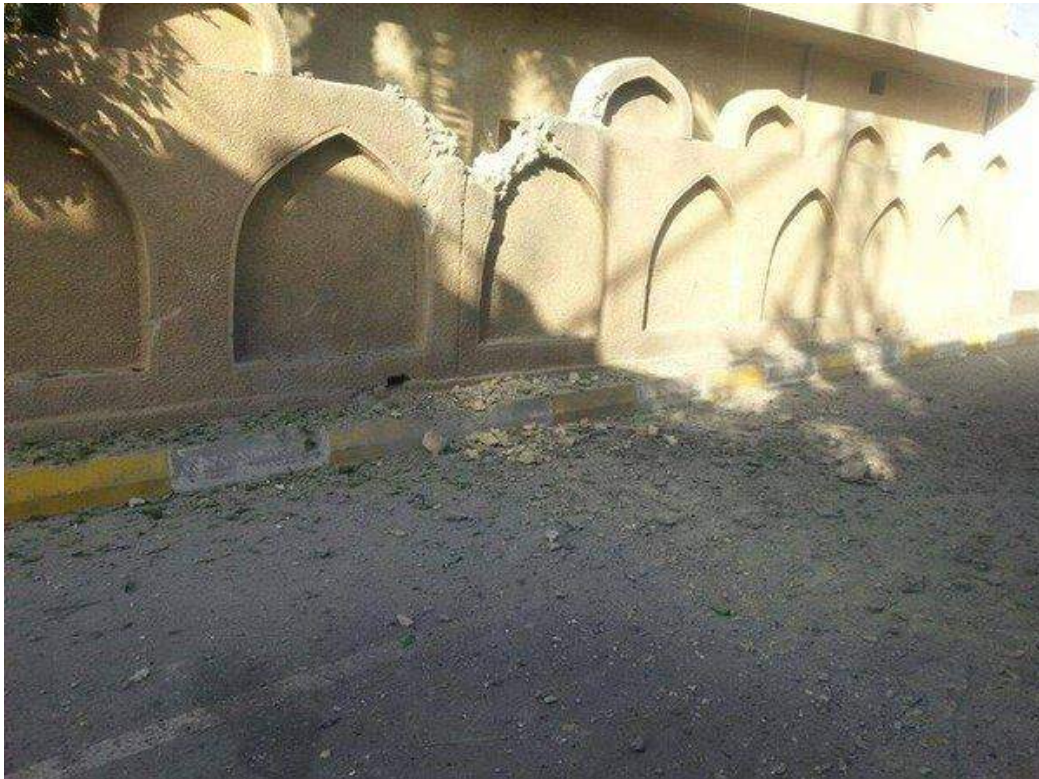
Damage to the exterior wall of al-Fayad Mosque (Twitter; November 15, 2014)
