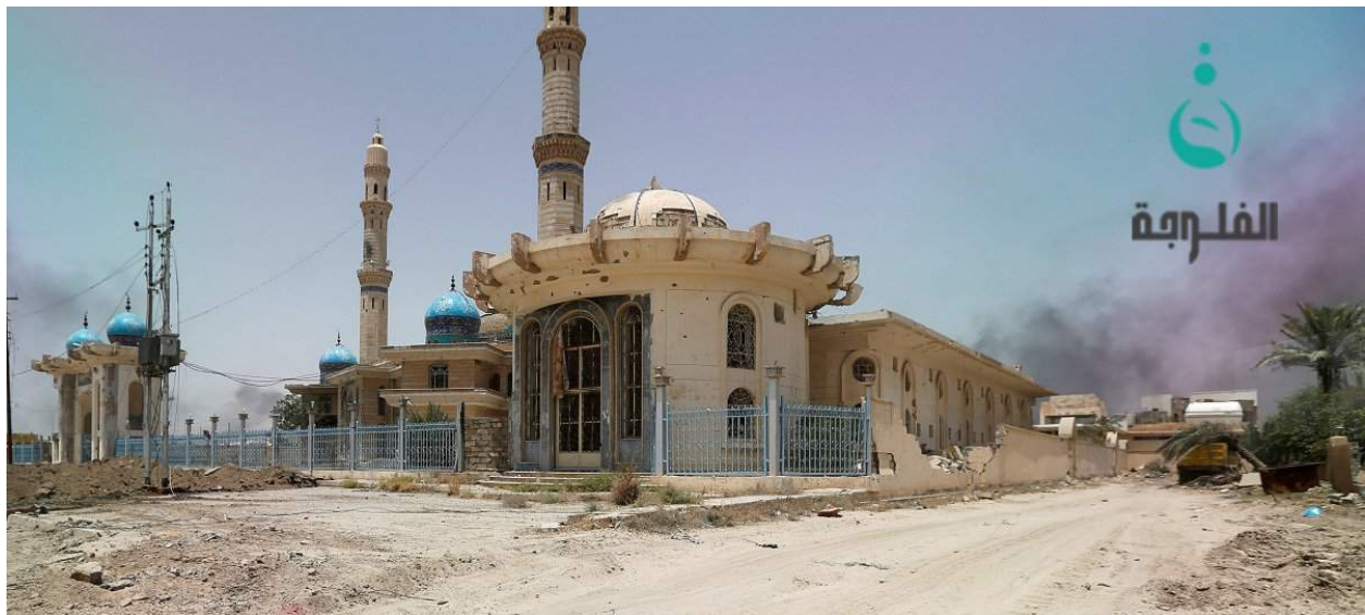
Damage to exterior of the Mosque of the Caliphs (Fallujah TV; June 20, 2016)
