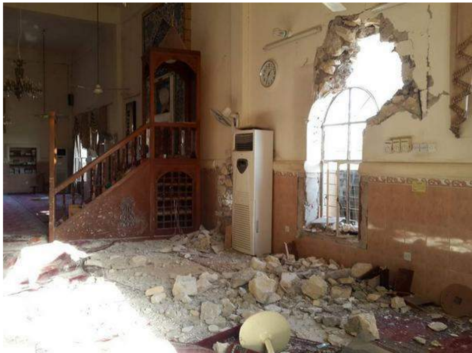
Damage and debris in interior of al-Sheikh Hamza Abbas Mosque (Iraq Now/Twitter; August 14, 2014)
