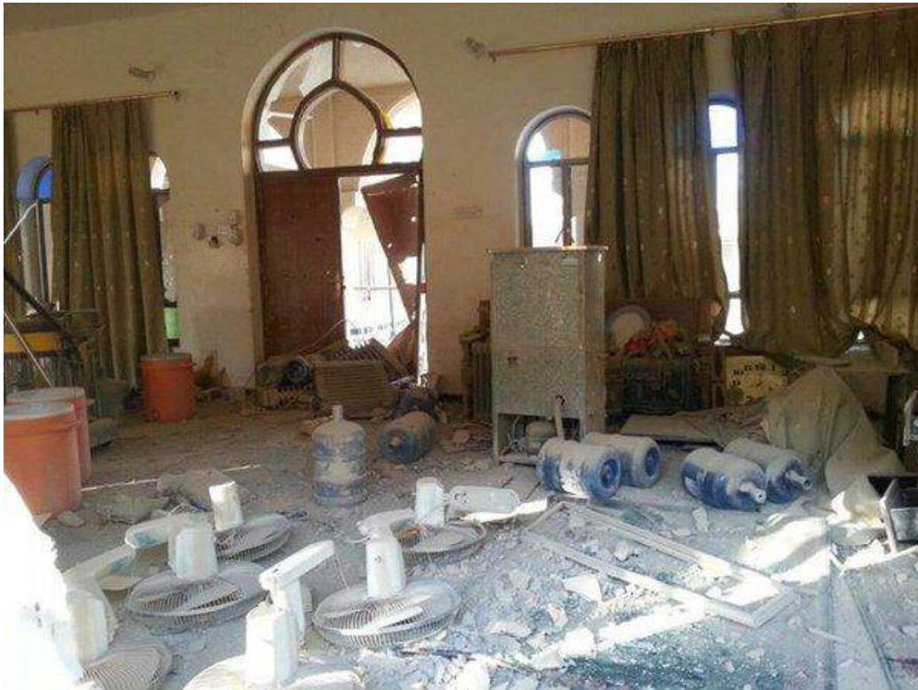
Damage and debris in the interior of al-Fayad Mosque (Twitter; November 15, 2014)
