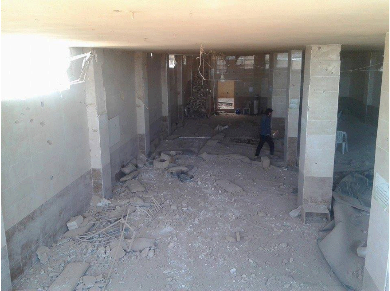
Damage to the interior of al-Foqani Mosque in Hbit (SNHR; June 28, 2016)
