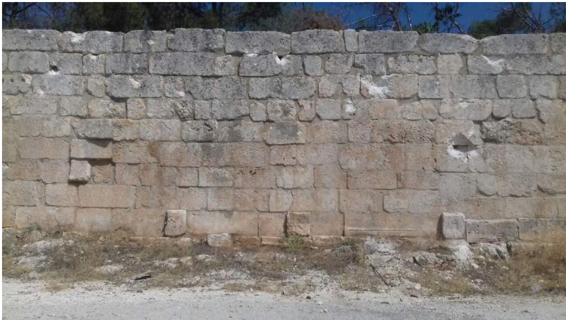
Damage to external wall, photo facing west
