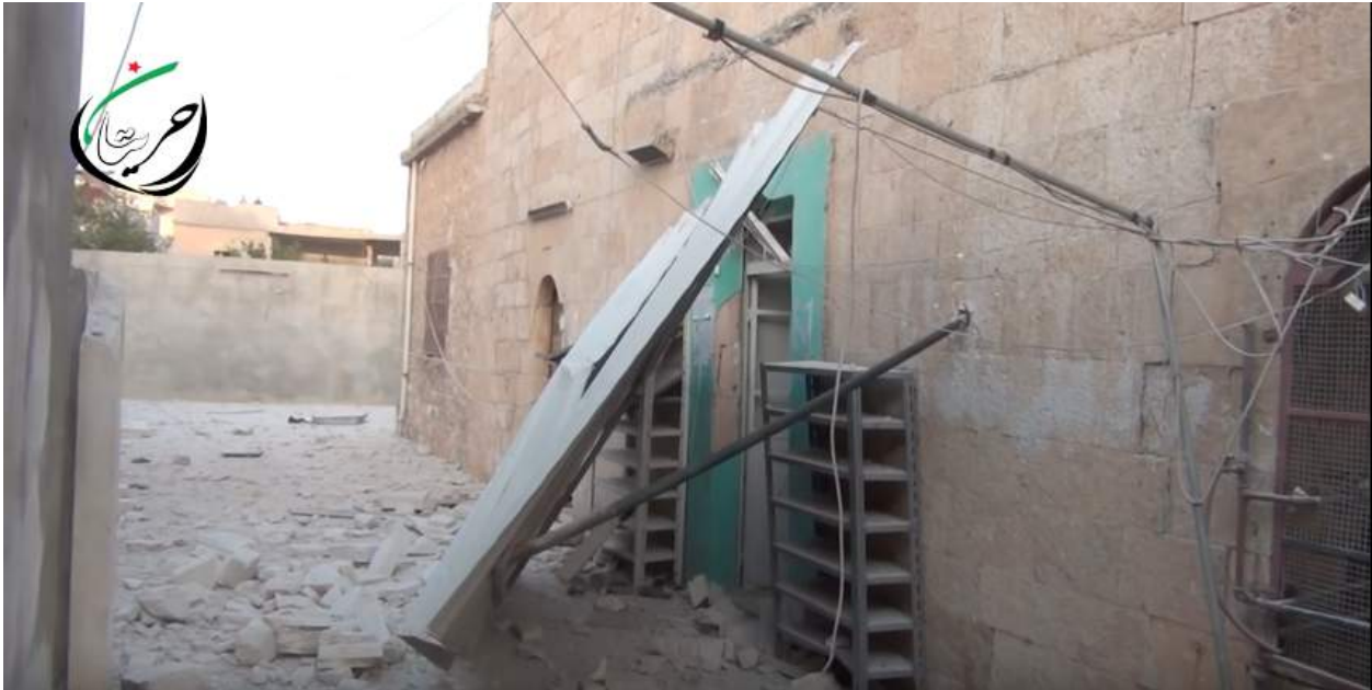
Video still of damage to the exterior of Khaled Bin al-Walid Mosque (Hraitan City; June 19, 2016)
