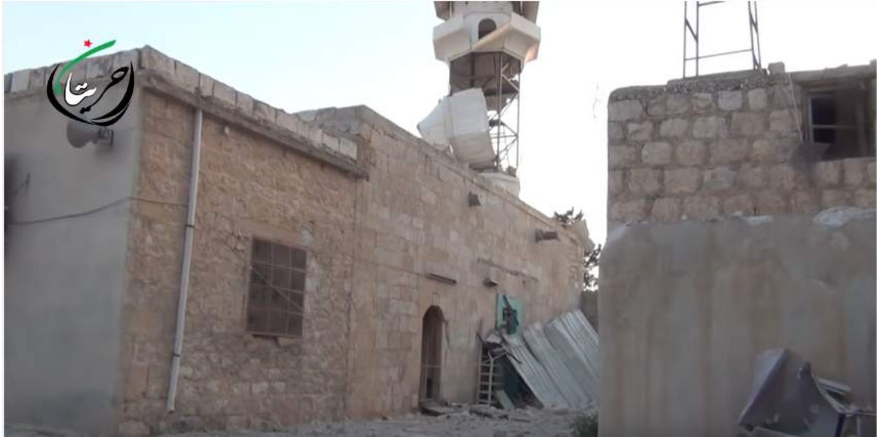
Video still of damage to the minaret of Khaled Bin al-Walid Mosque (Hraitan City; June 19, 2016)
