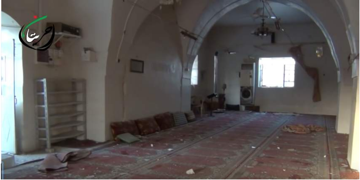
Video still of damage to the interior of Khaled Bin al-Walid Mosque (Hraitan City; June 19, 2016)
