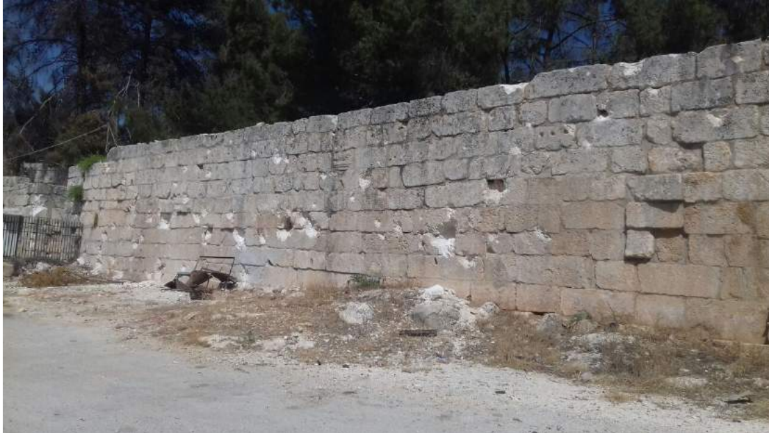
External wall damaged by shrapnel, photo facing southwest
