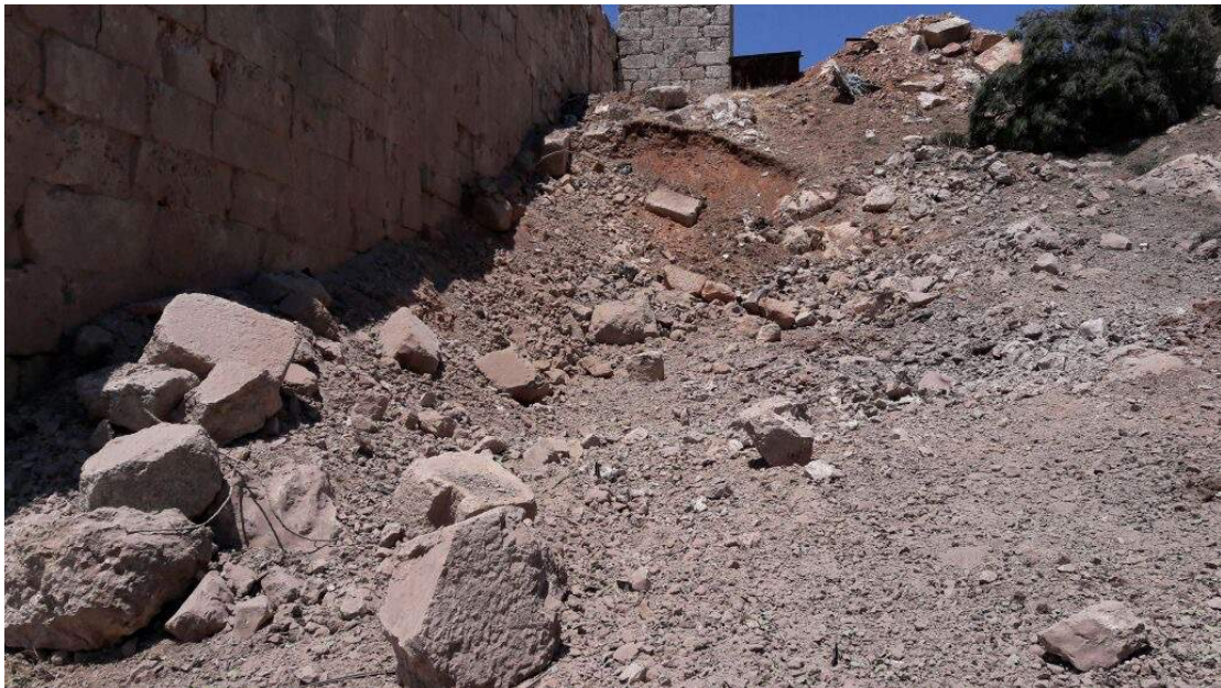
Damage to northeast outer wall
