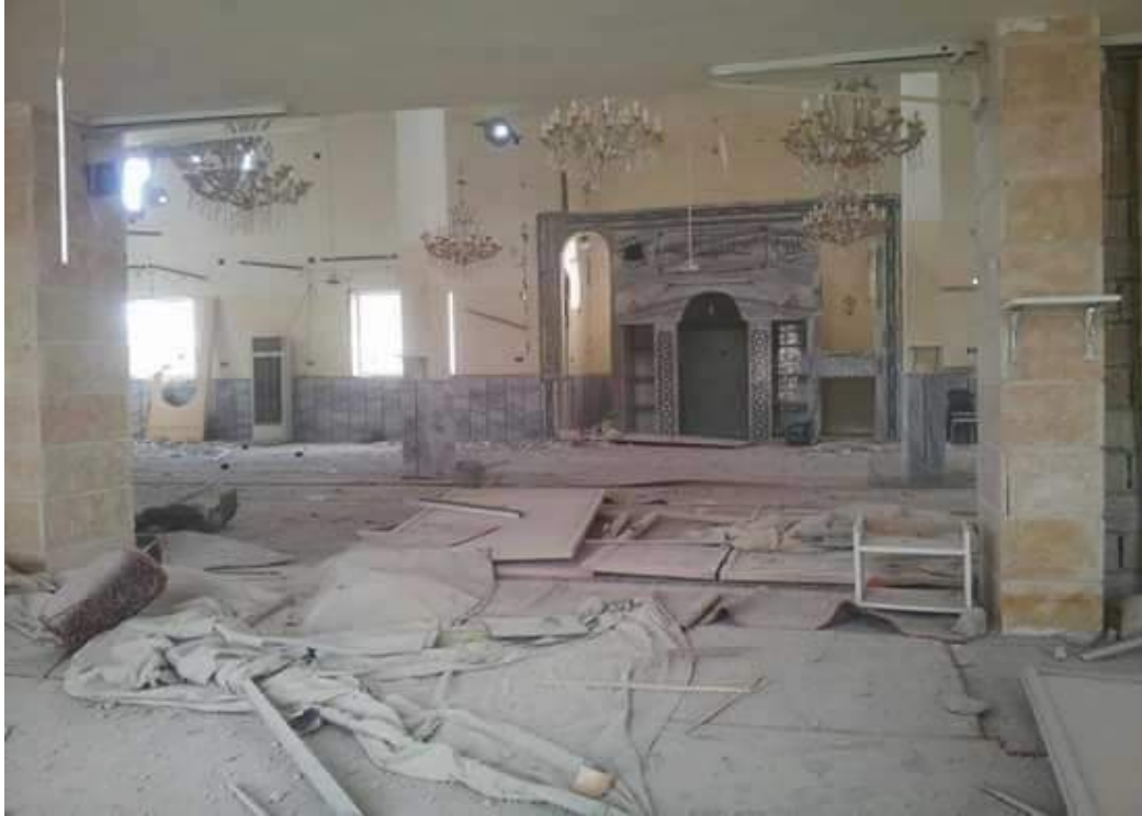
A photograph of what is likely damage to the interior of Bani Allou Mosque (Sukhna al-Hadath; May 28, 2016)
