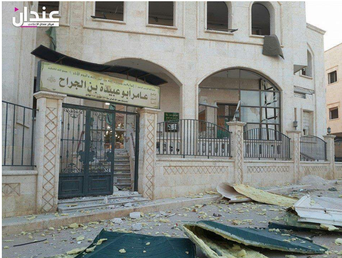
Damage to entrance of Amer Abu Obaida Ibn al-Jarah Mosque (Anadan Media Center; May 30, 2016)
