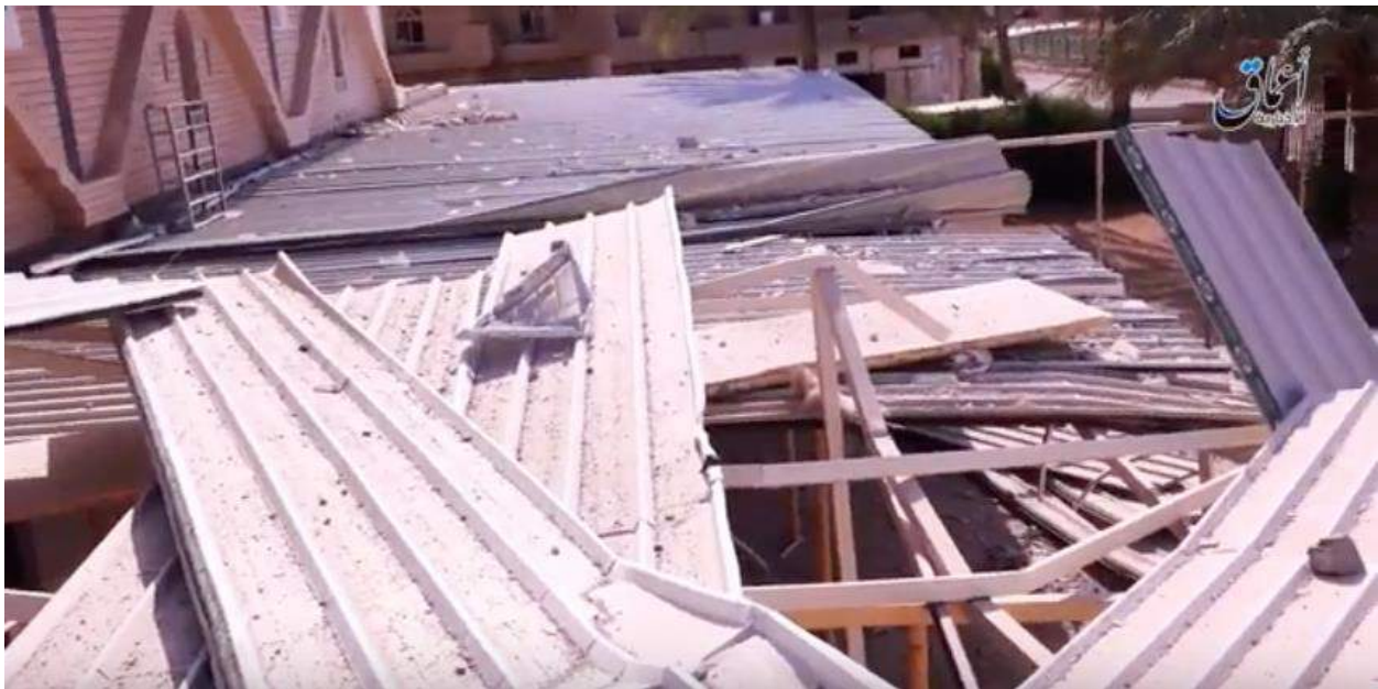
Video still of damage to al-Mudallal Mosque (Amaq News Agency; May 28, 2016)
