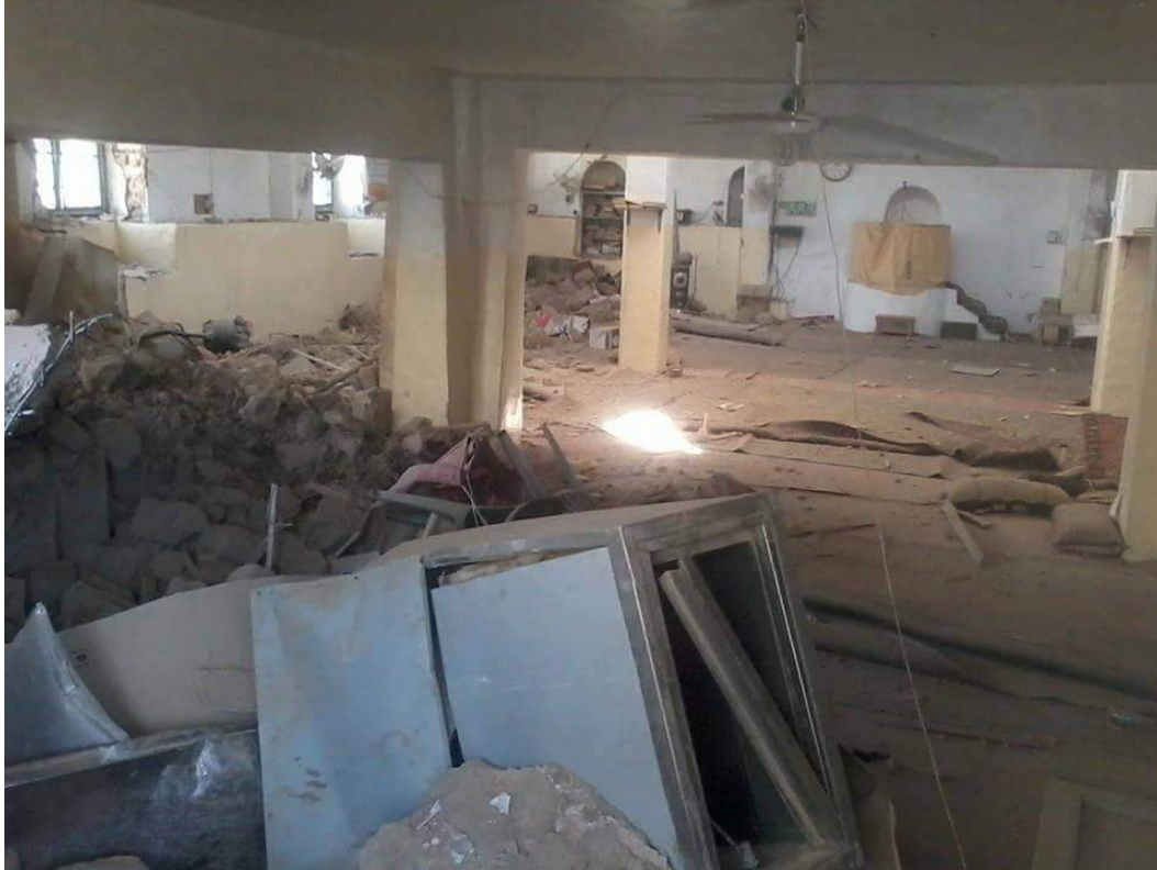
Interior damage to Uthman bin Affan Mosque (Sukhna al-Hadath; May 20, 2016)
