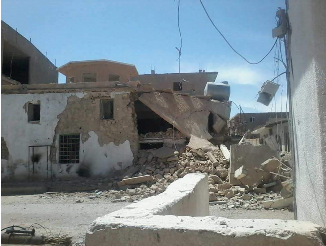
Exterior damage to Uthman bin Affan Mosque (Sukhna Al Hadath; May 20, 2016)
