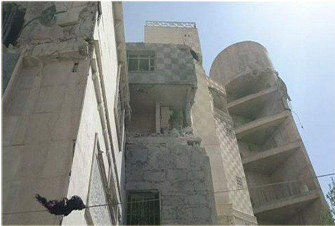
Exterior damage to al-Huda Mosque (AGPS; May 27, 2016)
