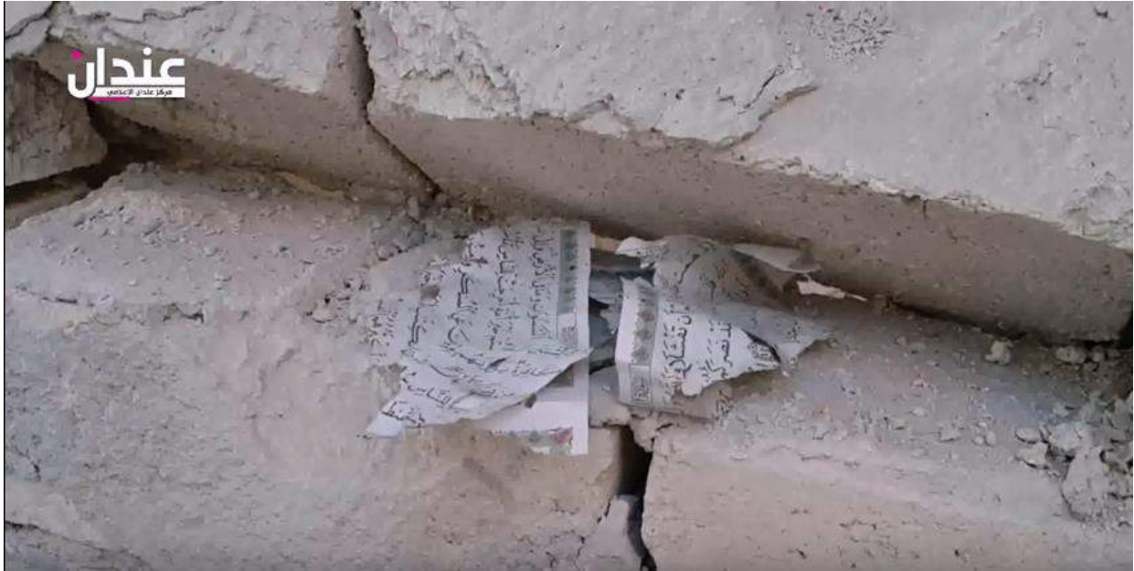
Video still of damage to Amer Abu Obaida Ibn al-Jarah Mosque (Anadan Media Center; May 30 2016)
