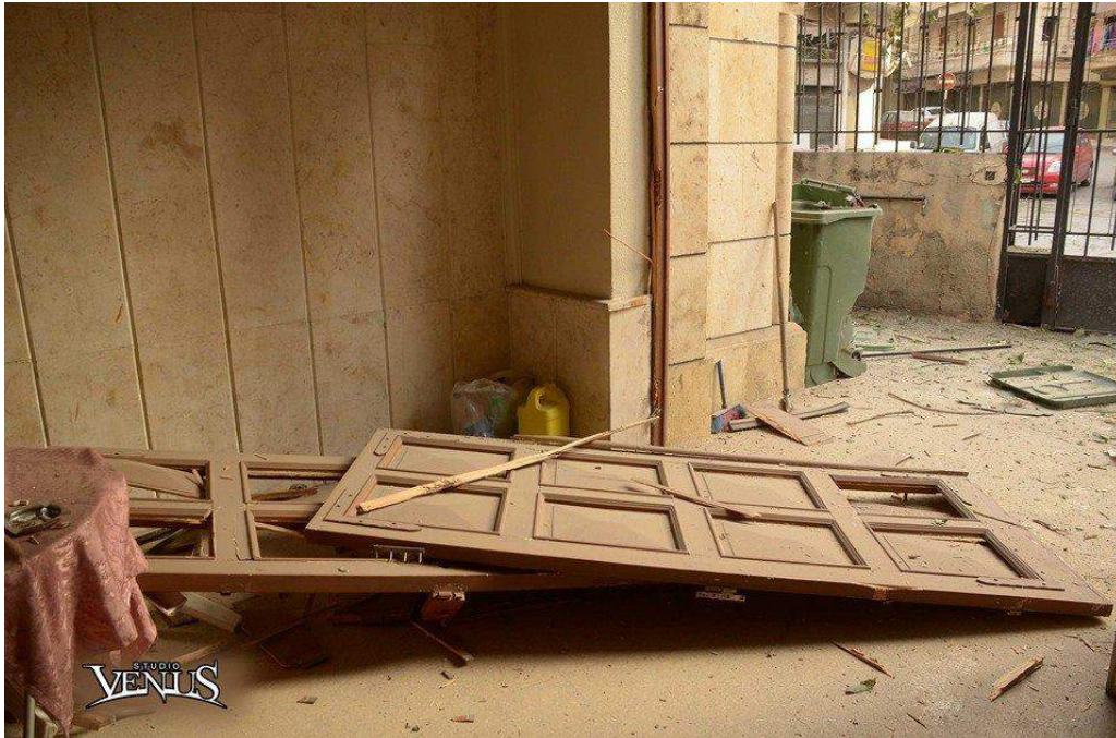
Damage to church doorway (Kantsasar/Studio Venus; June 5, 2016)
