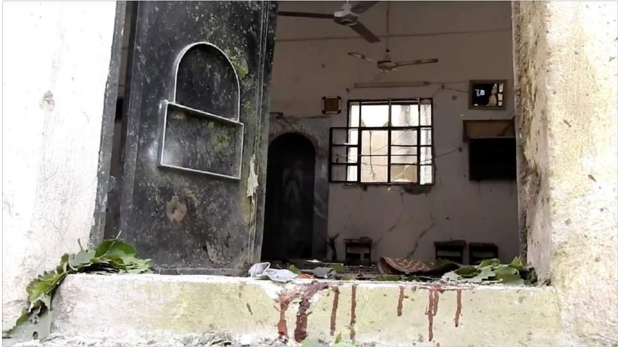
Video still of damage to the interior of Souq al-Hal Mosque (Ammar al-Nasser; May 9, 2016)
