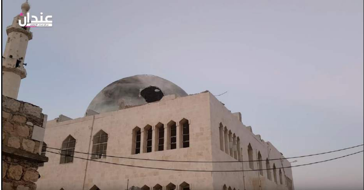
Video still of damage to the dome of Hamza bin Abdul Muttaleb Mosque (Anadan Media Center; May 31, 2016)
