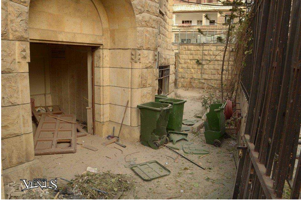
Damage to an entrance of the church (Kantsasar/Studio Venus; June 5, 2016)
