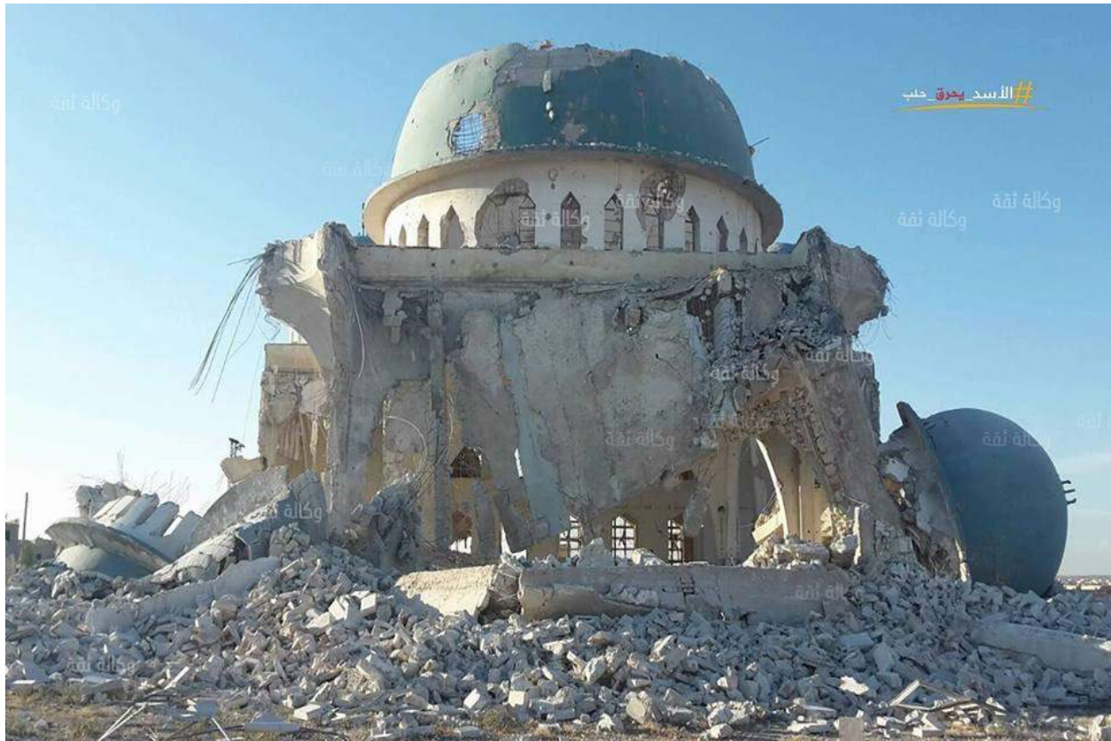
Extensive damage to Sahib bin Sinan al-Roumi Mosque, including the destruction of at least two of the domes (Khaled Al Homsî; June 7, 2016)
