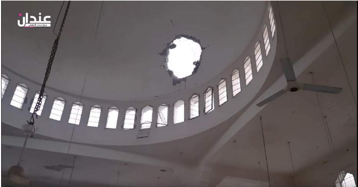
Video still of damage to the dome of Hamza bin Abdul Muttaleb Mosque (Anadan Media Center; May 31, 2016)
