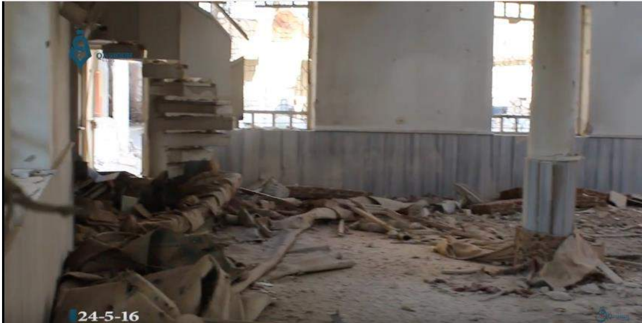
Video still of damage to the interior, including a staircase, of al-Kabir Mosque (Qasioun News Agency; May 24, 2016)
