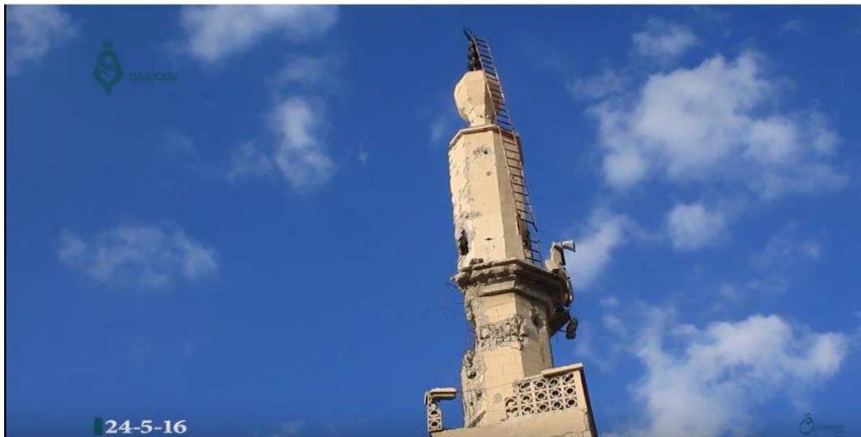
Video still of the damaged minaret of al-Kabir Mosque (Qasioun News Agency; May 24, 2016)
