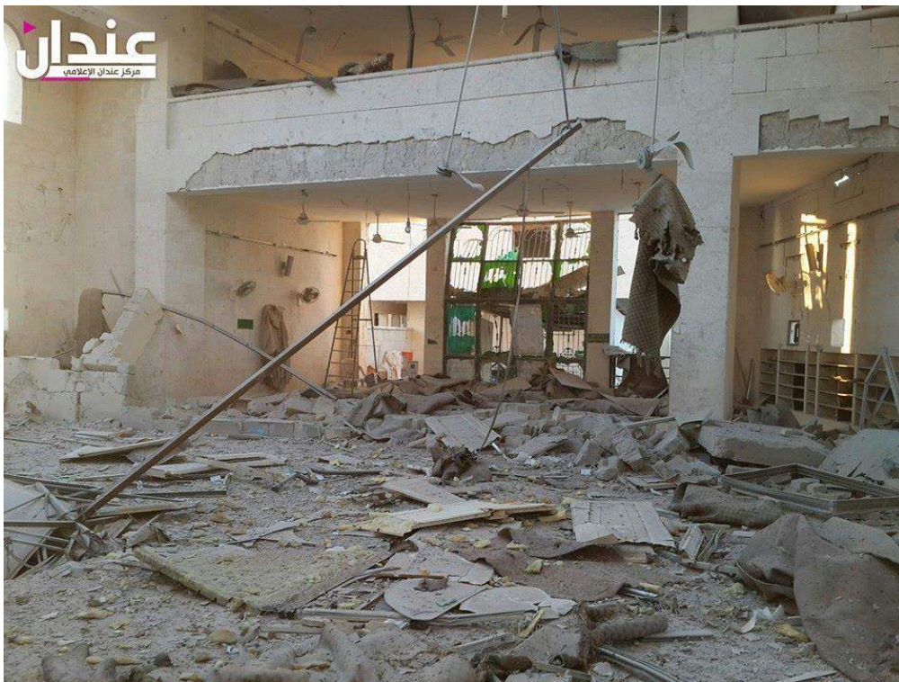
Damage to the interior of Amer Abu Obaida Ibn al-Jarah Mosque (Anadan Media Center; May 30, 2016)
