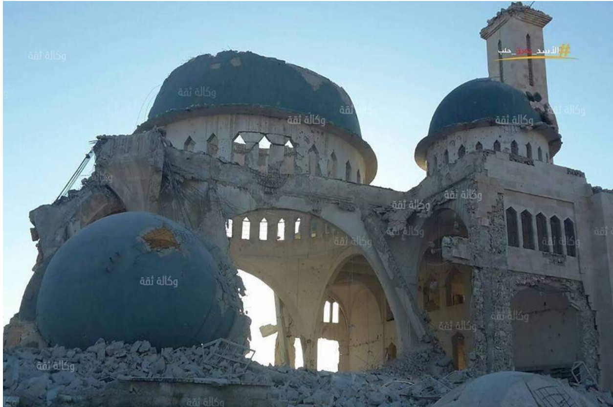
Damage to Sahib bin Sinan al-Roumi Mosque, showing extensive damage to the building, domes, and minarets (Khaled Al Homsy; June 7, 2016)
