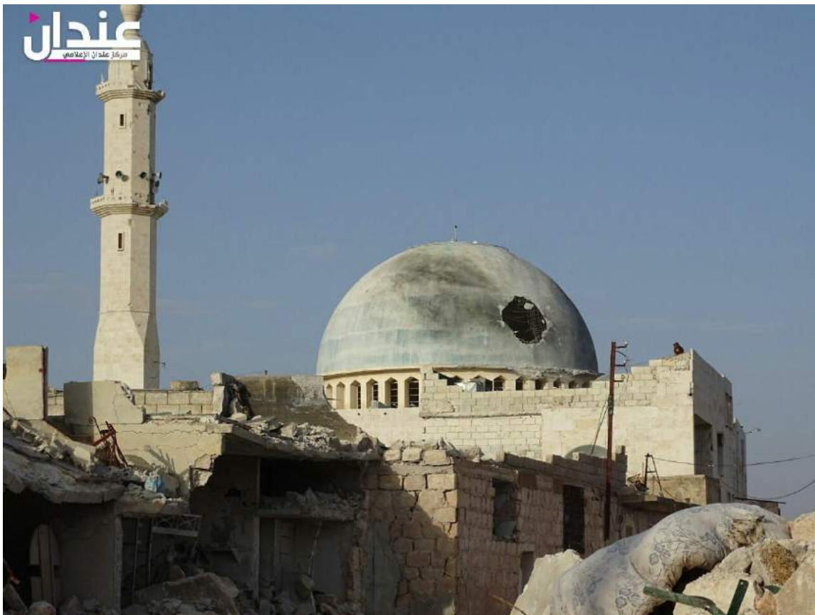
Damage to dome and exterior of Hamza bin Abdul Muttaleb Mosque (SNHR; May 31, 2016)
