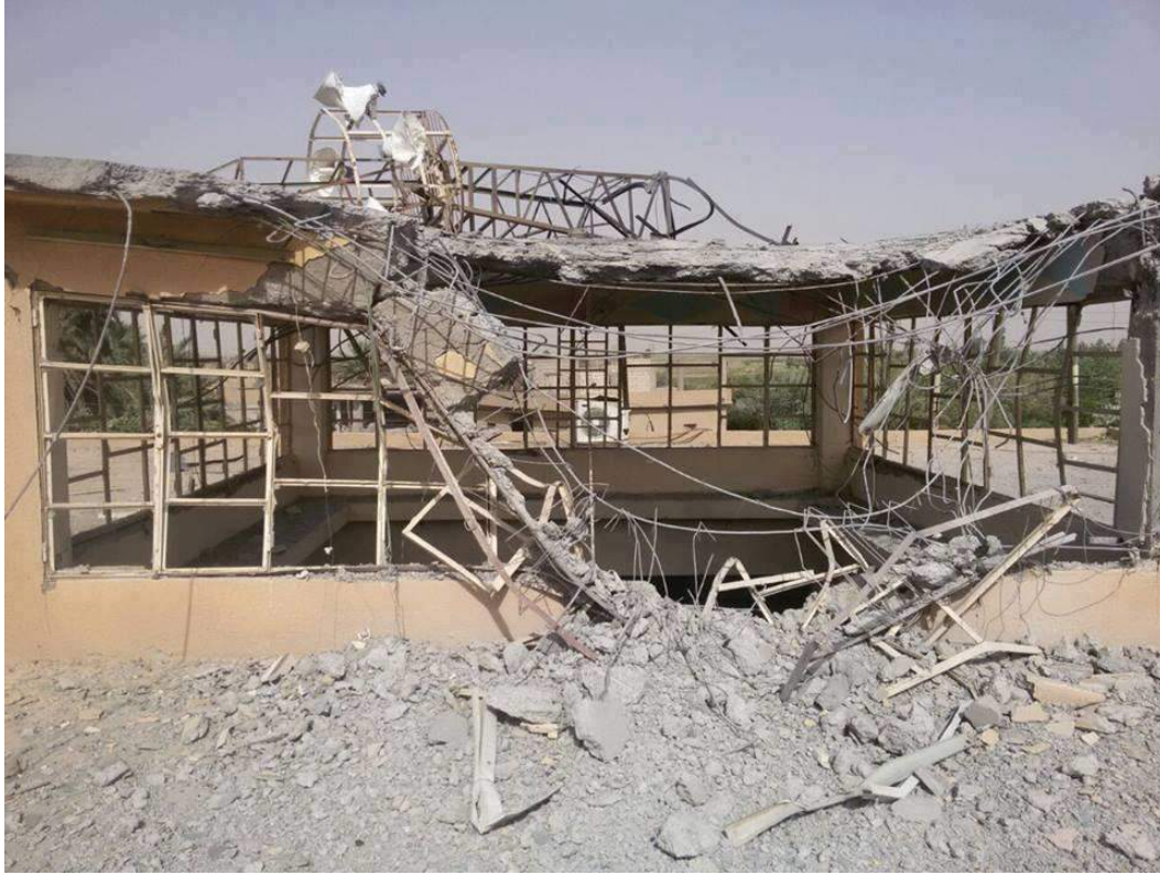
Damage to Abu Bakr al-Sadeiq Mosque (SNHR; June 3, 2016)
