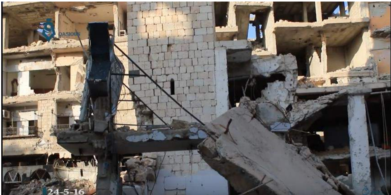
Video still of damage to al-Kabir Mosque (Qasioun News Agency; May 24, 2016)
