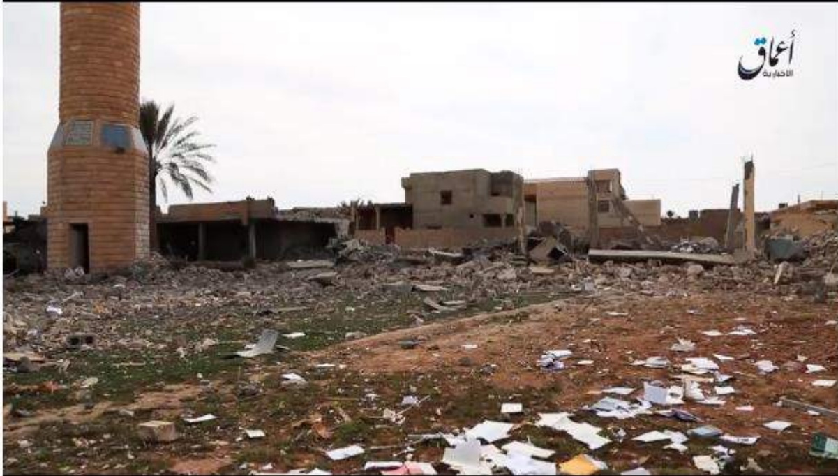
Still image of the damage to the surrounding area of al-Farooq Mosque (Internet Archive; March 15, 2016)
