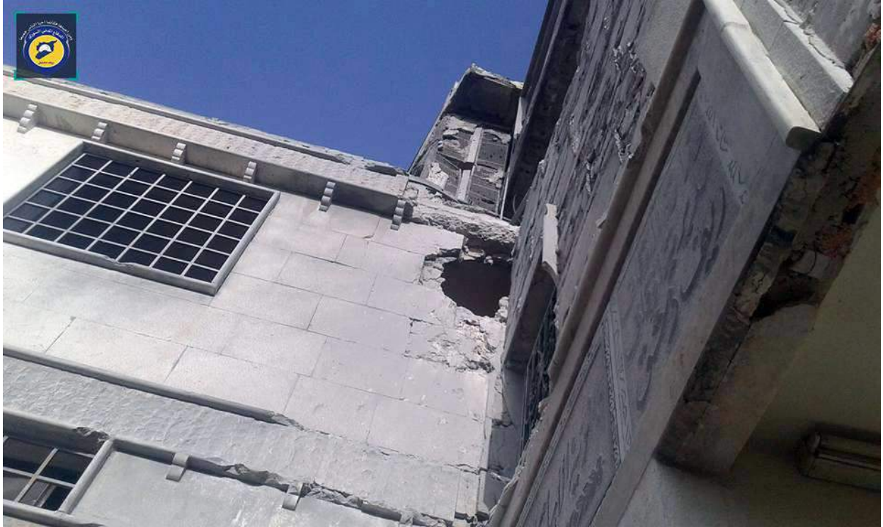
Exterior damage to al-Huda Mosque, including a medium-sized hole in one wall of the mosque (The White Helmets, Rif Dimashq; May 27, 2016)
