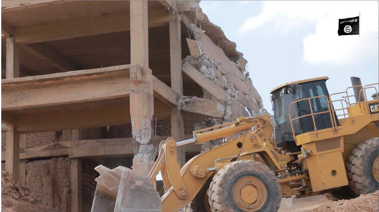
Video still of an earthmover driving into the reconstructed Adad Gate (Amaq News Agency; Downloaded June 7, 2016)
