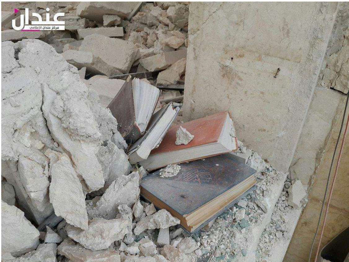
Video still of damage to Amer Abu Obaida Ibn al-Jarah Mosque (Anadan Media Center; May 30, 2016)
