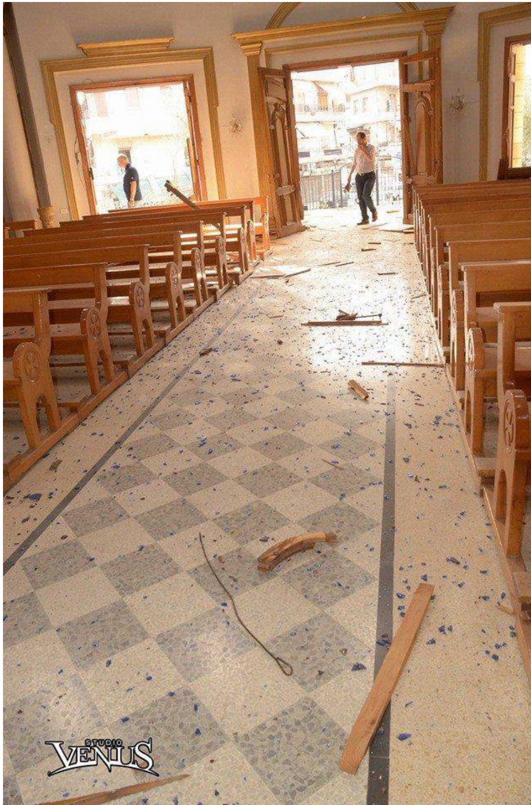
Damage and debris in church interior (Kantsasar/Studio Venus; June 5, 2016)
