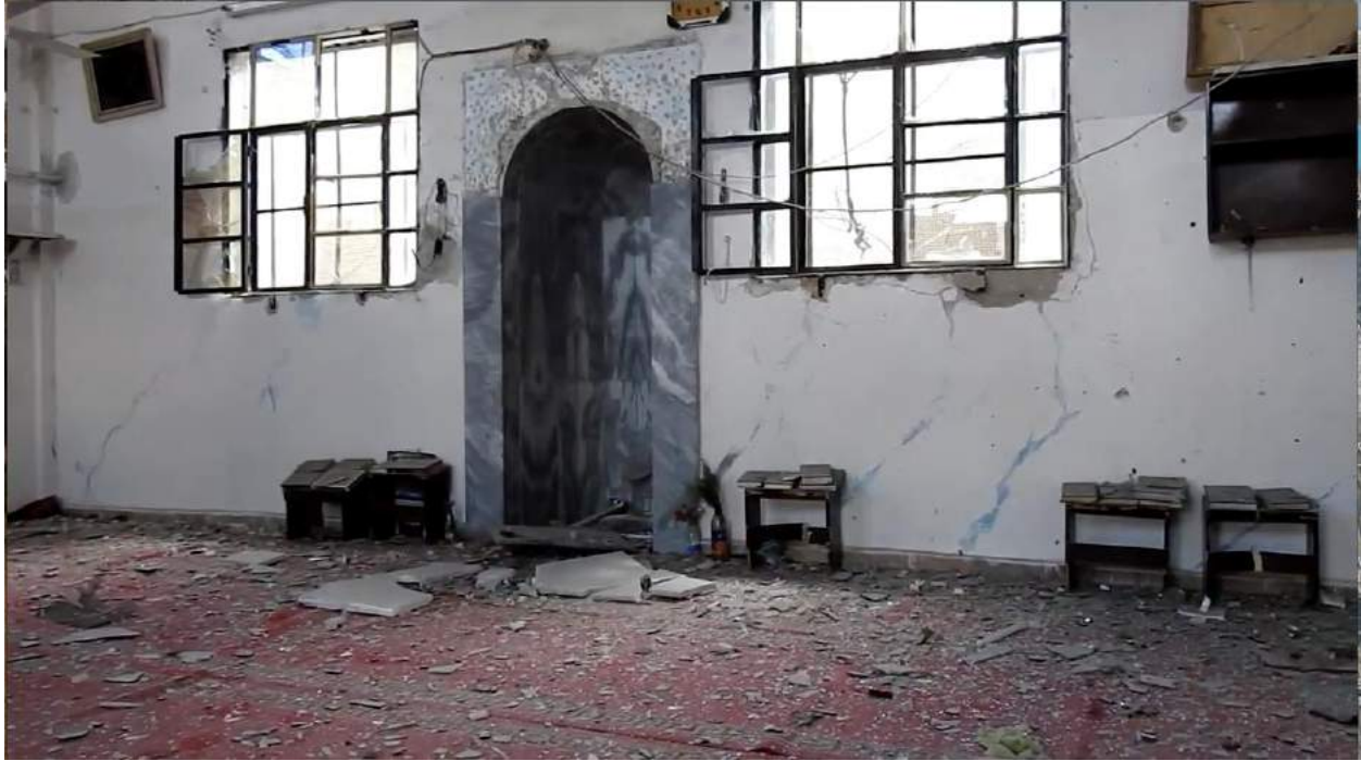
Video still of damage to the interior of Souq al-Hal Mosque (Ammar al-Nasser; May 9, 2016)
