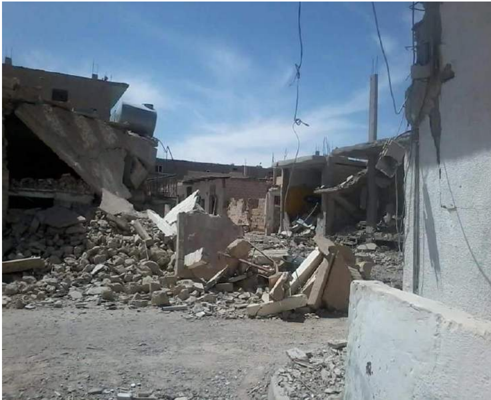
Surrounding damage at Uthman bin Affan Mosque (Sukhna al-Hadath; May 20, 2016)
