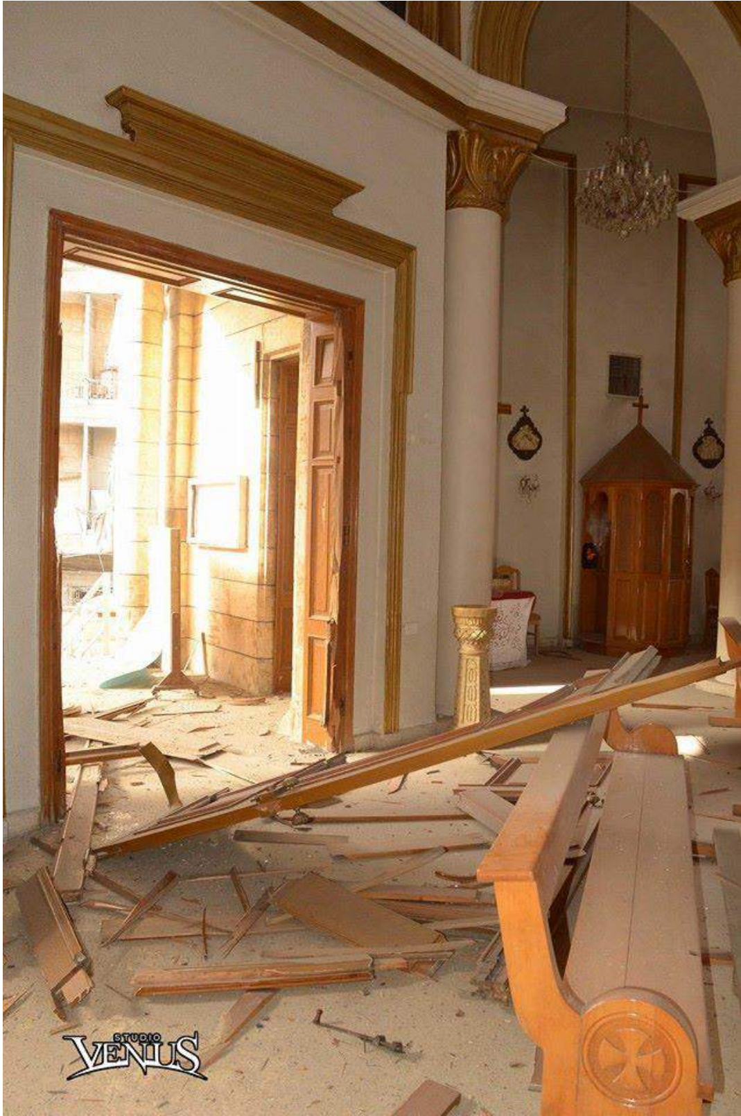
Damage to church doorway and pews (Kantsasar/Studio Venus; June 5, 2016)
