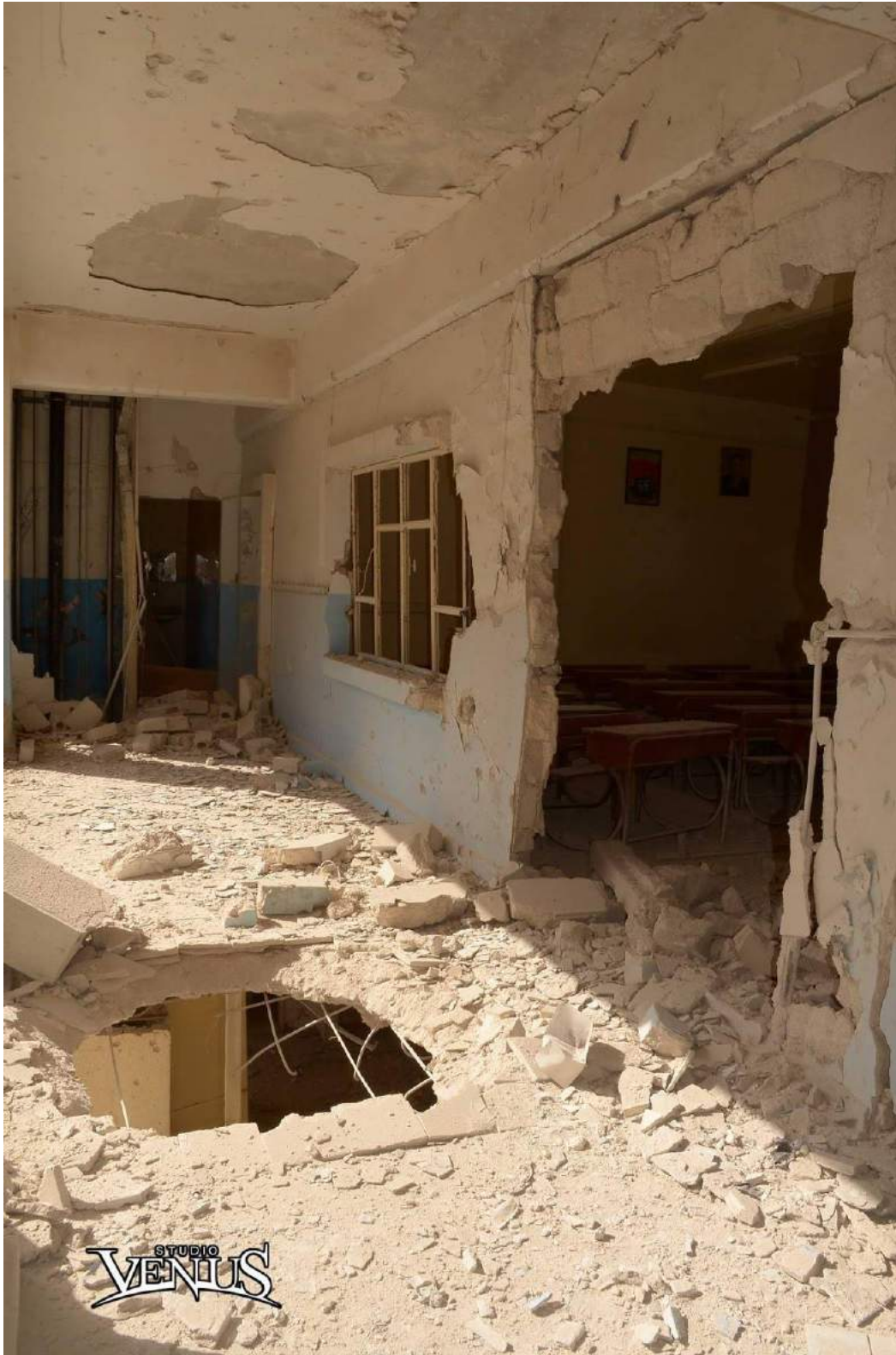
Damage to Zvartnots School classroom (Kantsasar/Studio Venus; June 3, 2016)
