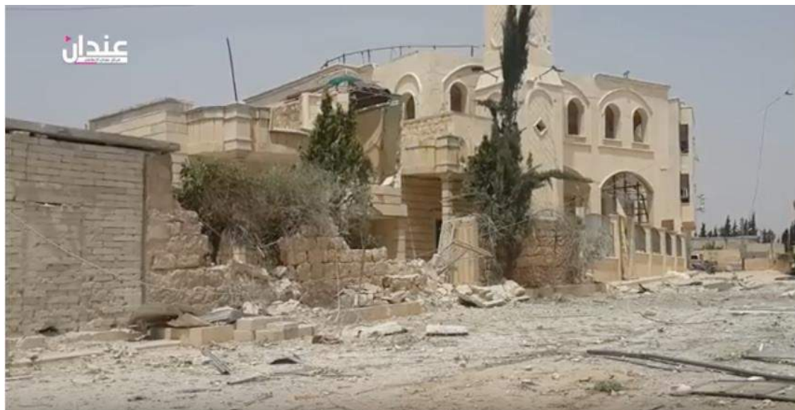
Video still of damage to exterior of Amer Abu Obaida Ibn al-Jarah Mosque (Anadan Media Center; June 3, 2016e)
