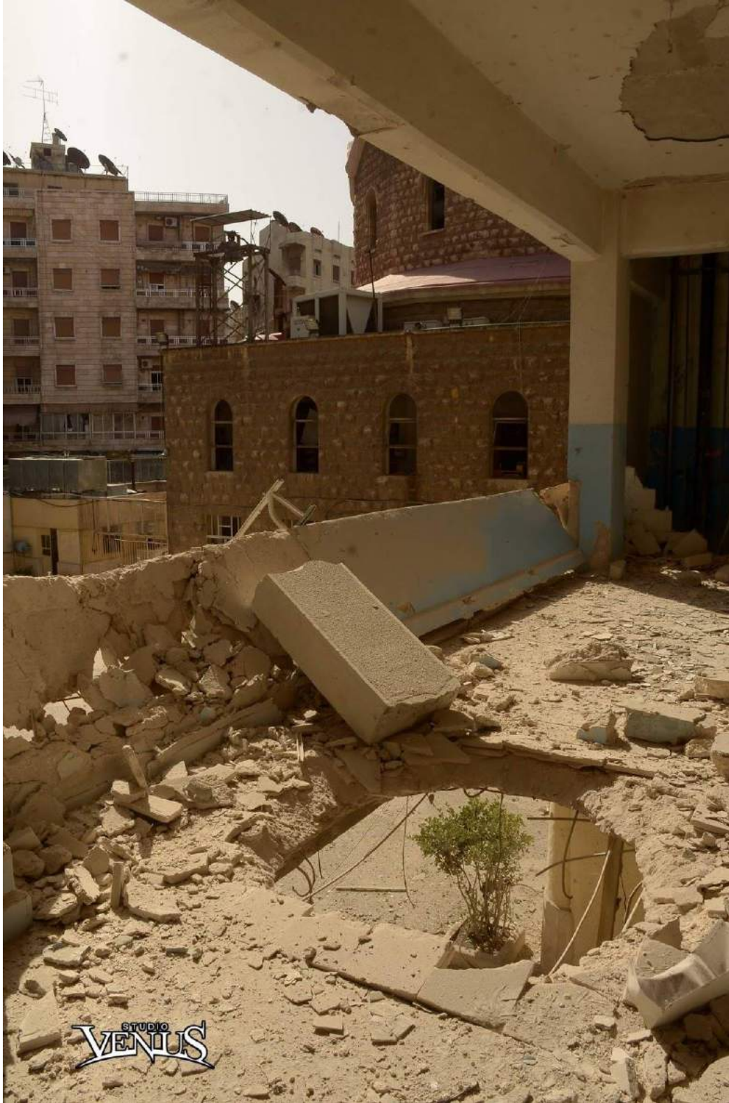
Severe structural damage to Zvartnots School (Kantsasar/Studio Venus; June 3, 2016)
