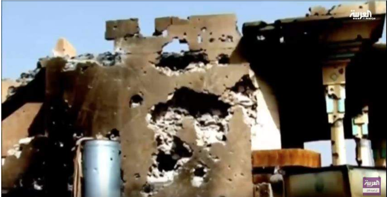
Video still of damage to one of the mosques allegedly damaged by the Popular Mobilization Front (Al Arabiya; May 28, 2016)
