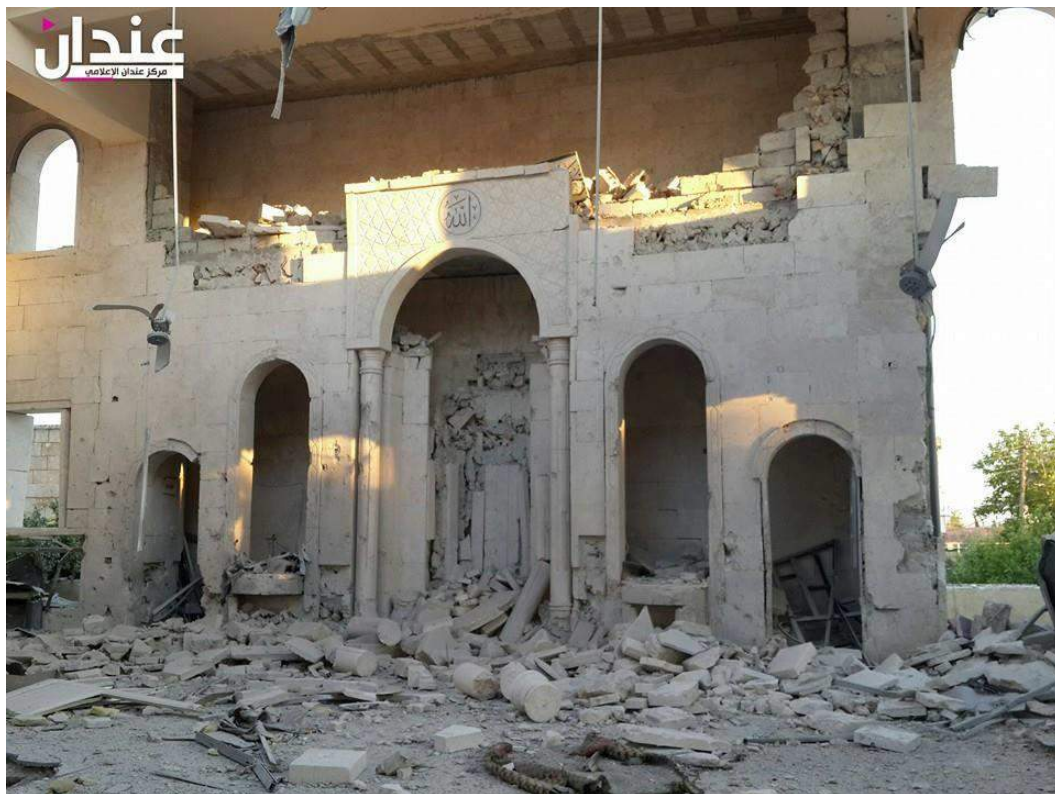
Damage to exterior of Amer Abu Obaida Ibn al-Jarah Mosque (SNHR; May 30, 2016)
