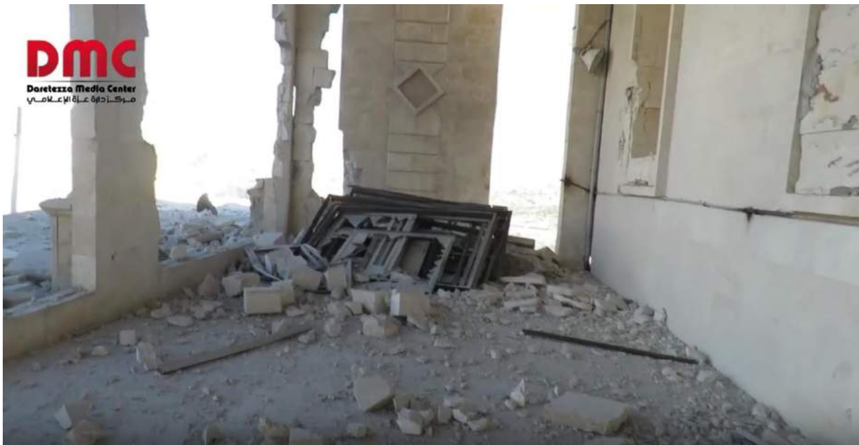
Video still showing damage to eastern side of al-Farouq Mosque (Daretezza Media Center; June 5, 2016)
