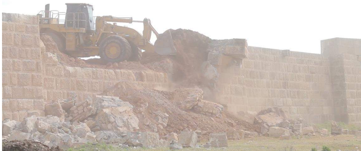
Video still of an earthmover demolishing Nineveh's reconstructed city wall, likely near the Mashki Gate (Amaq News Agency; Downloaded June 7, 2016)
