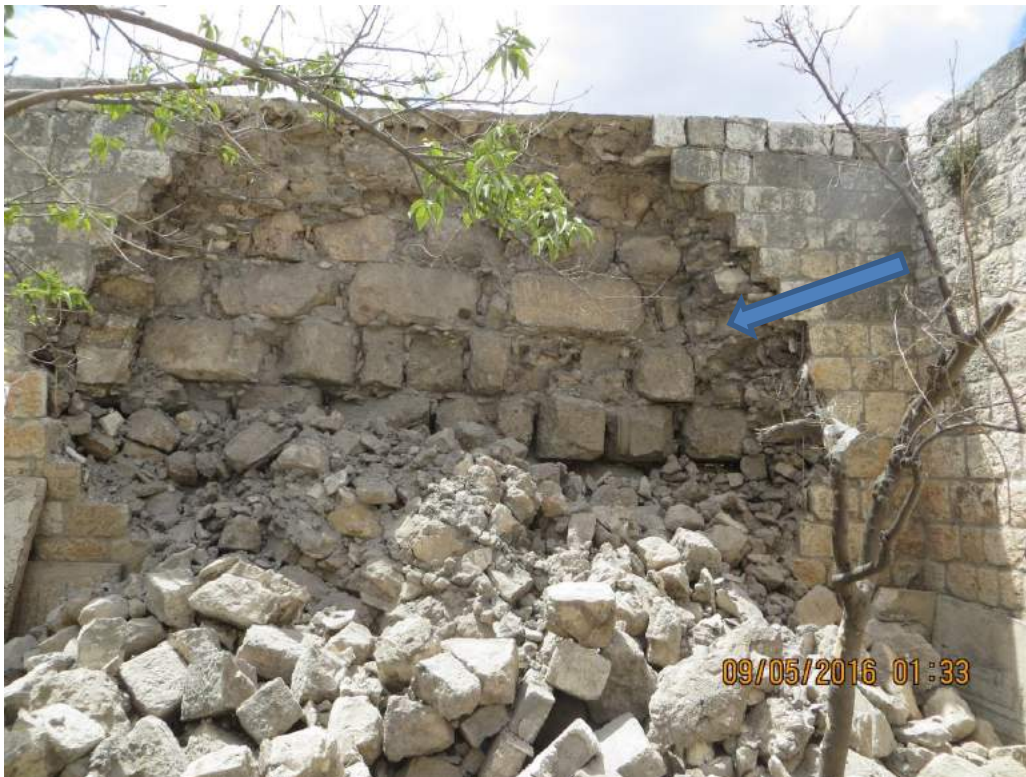
Damage to external wall (see plan above)
