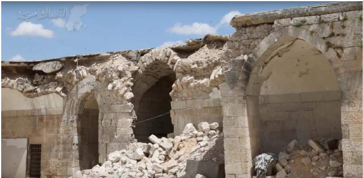
Video still of damage to the Al-Ma'arra Museum (El-Dorar Al Shami; May 9, 2016)
