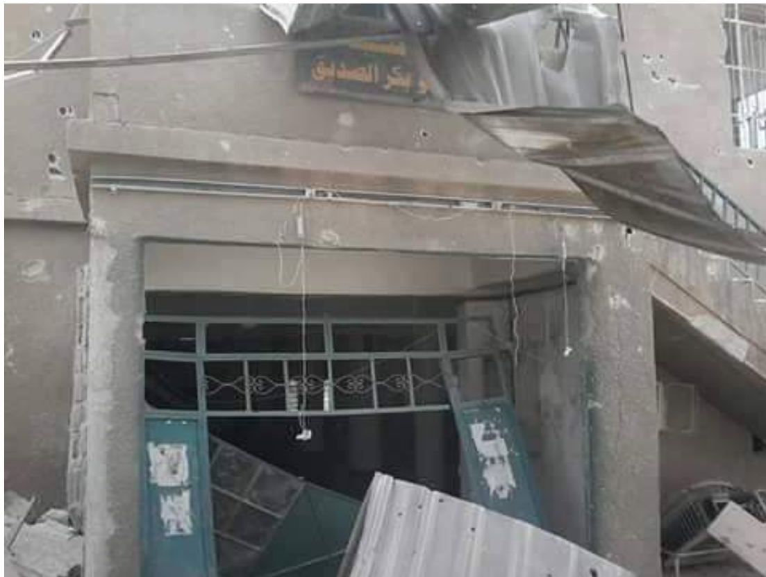
Damage to the entrance of the Abu Bakr al-Sidiq Mosque (SNHR; May 11, 2016)
