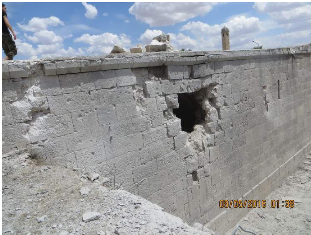
Damage causing a breach in the wall (outside)
