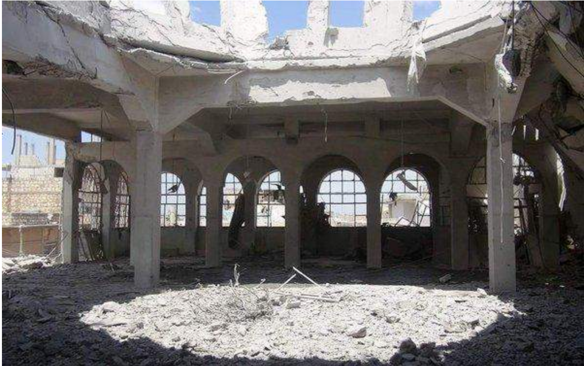
Light shines through where the dome once stood at Sheikh Shuayab Mosque (DOAM; May 10, 2016)
