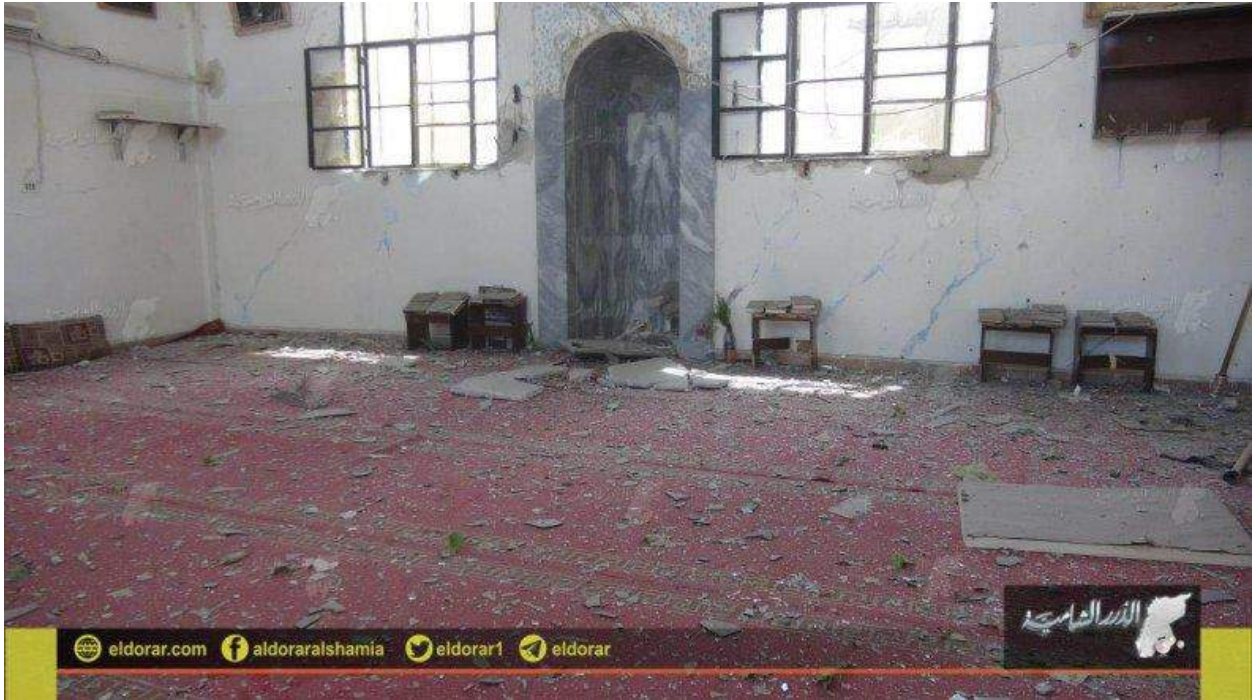
Possible image of interior damage to Al-Johari Mosque (El Dorar al-Shamia; May 9, 2016)
