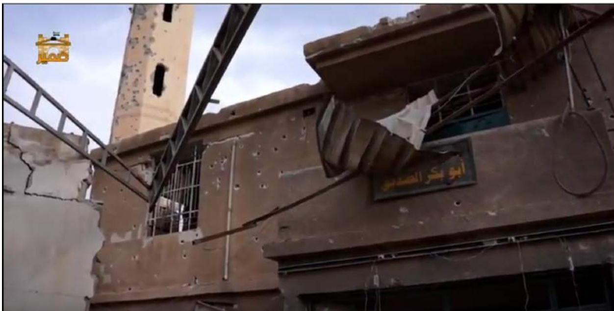
Damage to the exterior of the Abu Bakr al-Sidiq Mosque (Media Abu Mohammad; April 28, 2016)
