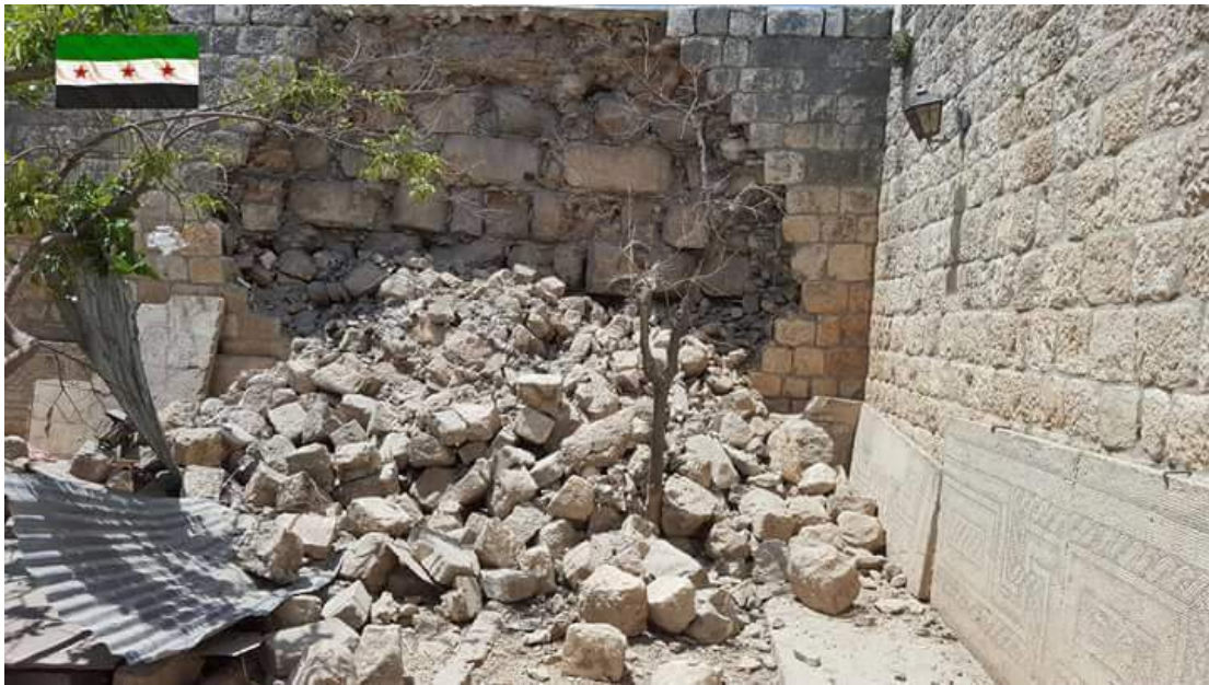
A crumbled exterior wall at the Al-Ma'arra Museum (Republished by APSA; May 9, 2016)
