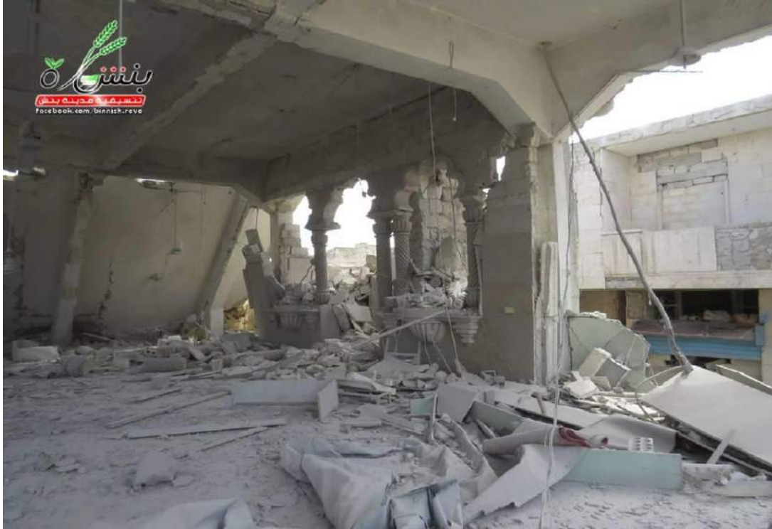
Interior damage at Sheikh Shuayab Mosque (Coordinators of the Revolution in the city of Binnish; May 10, 2016)
