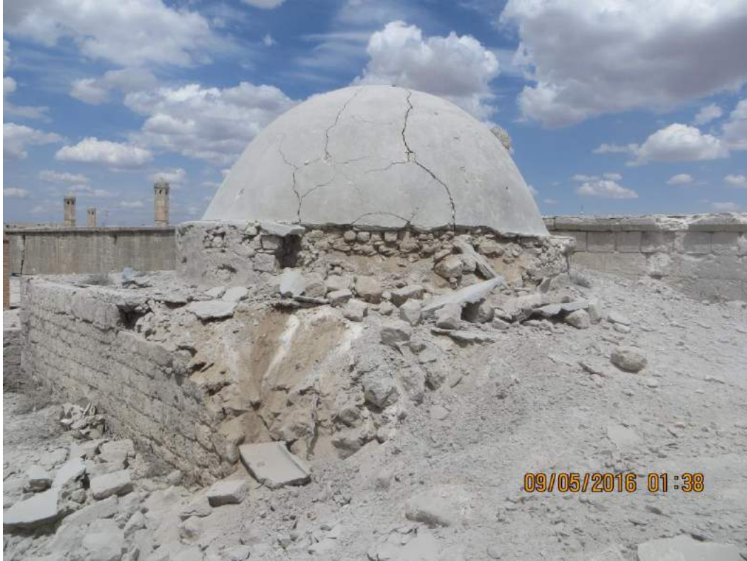
Damage to the main dome on the Bathhouse (Hammam) roof
