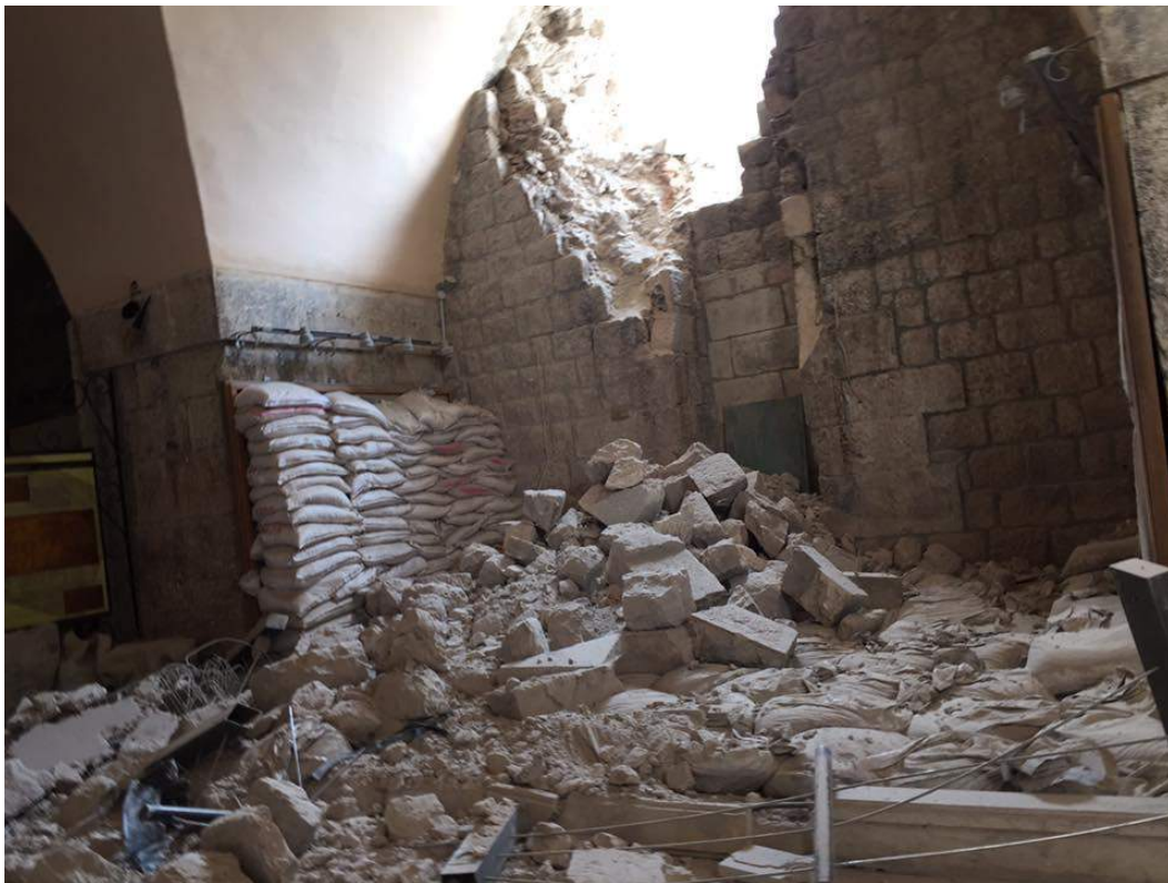
Airstrike damage to the Al-Ma'arra Museum (Al Watan FM; May 9, 2015)
