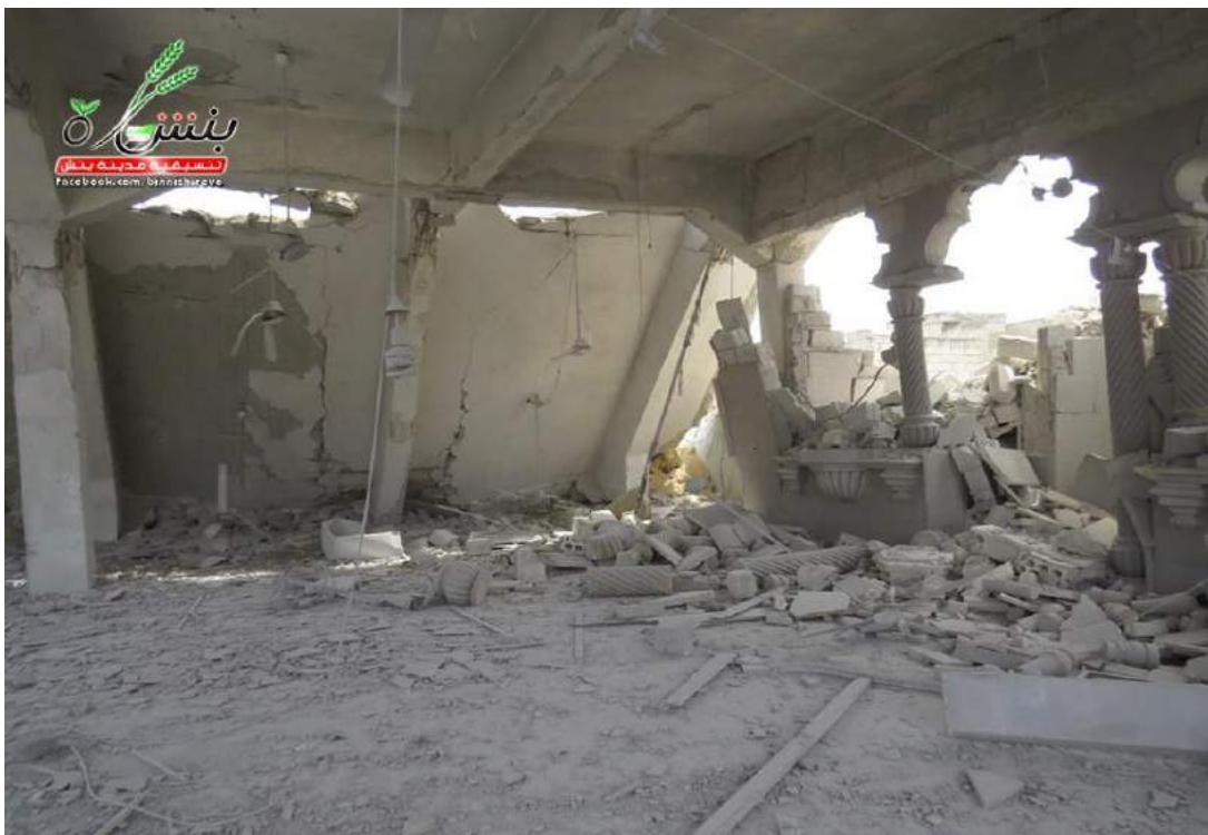
Interior damage to Sheikh Shuayab Mosque showing crumbling and partial wall collapse (Coordinators of the Revolution in the city of Binnish; May 10, 2016)
