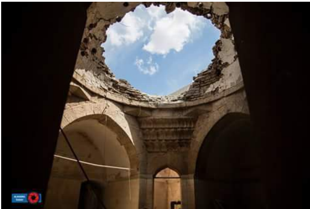
Damage to the dome at the Al-Ma'arra Museum (Al Marra Today; May 9, 2016)
