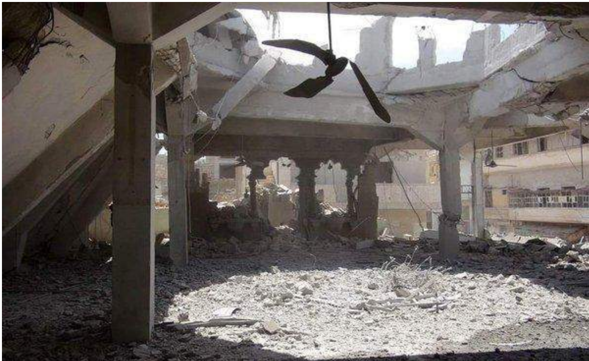
Interior damage to Sheikh Shuayab Mosque (DOAM; May 10, 2016)
