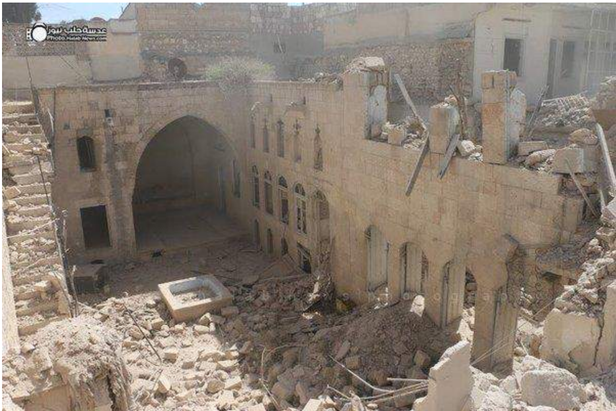
Severe damage to the Nabhaniyah Institute (Twitter; April 29, 2016)
