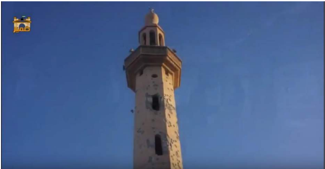
Detail of damage to the minaret (Media Abu Mohammad; April 28, 2016)
