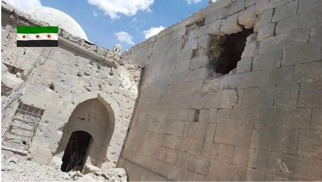
Airstrike damage to the Al-Ma'arra Museum (Republished by APSA; May 9, 2016)
