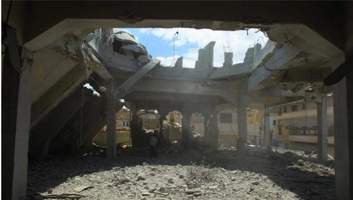
Interior damage to Sheikh Shuayab Mosque (Al Jazeera/Reuters; May 10, 2016)
