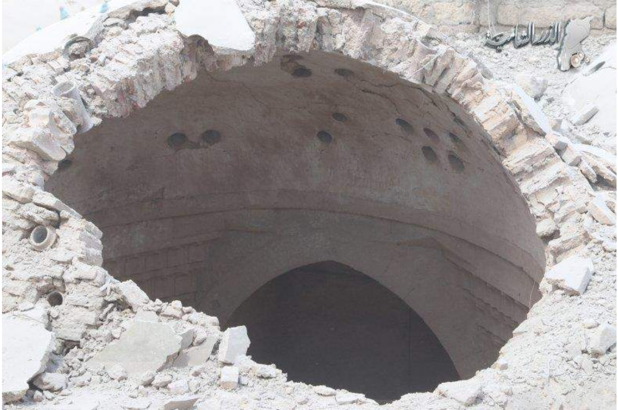
Damage to the dome of the Al-Ma'arra Museum (El-Dorar Al Shami; May 9, 2016)
