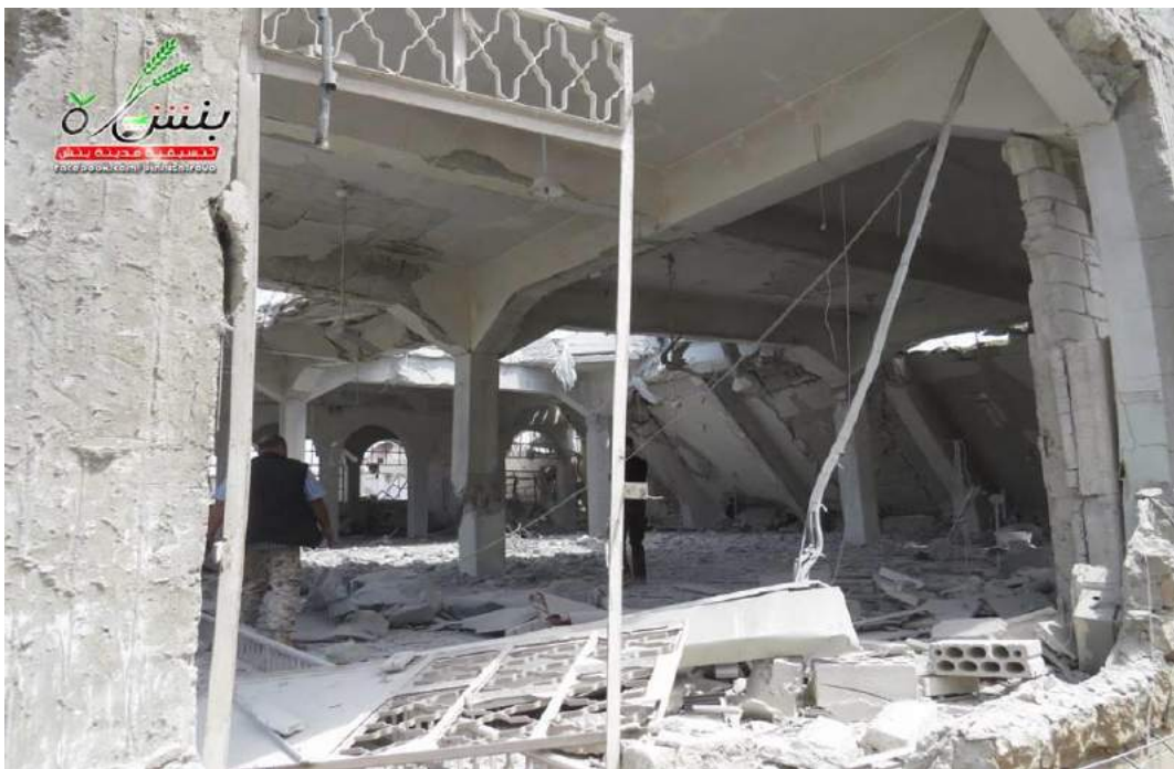
Photograph of interior damage to Sheikh Shuayab Mosque (Coordinators of the Revolution in the city of Binnish; May 10, 2016)
