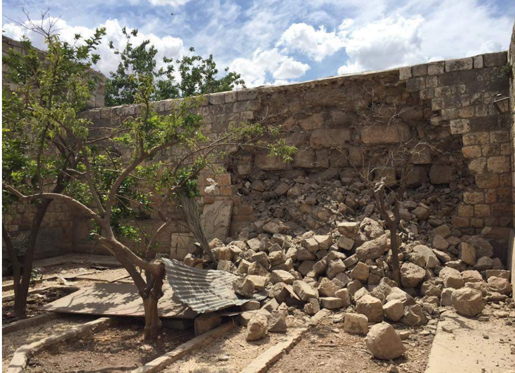
Damage to exterior wall of the Al-Ma'arra Museum Al-Ma'arra Museum (Al Watan FM; May 9, 2015)
