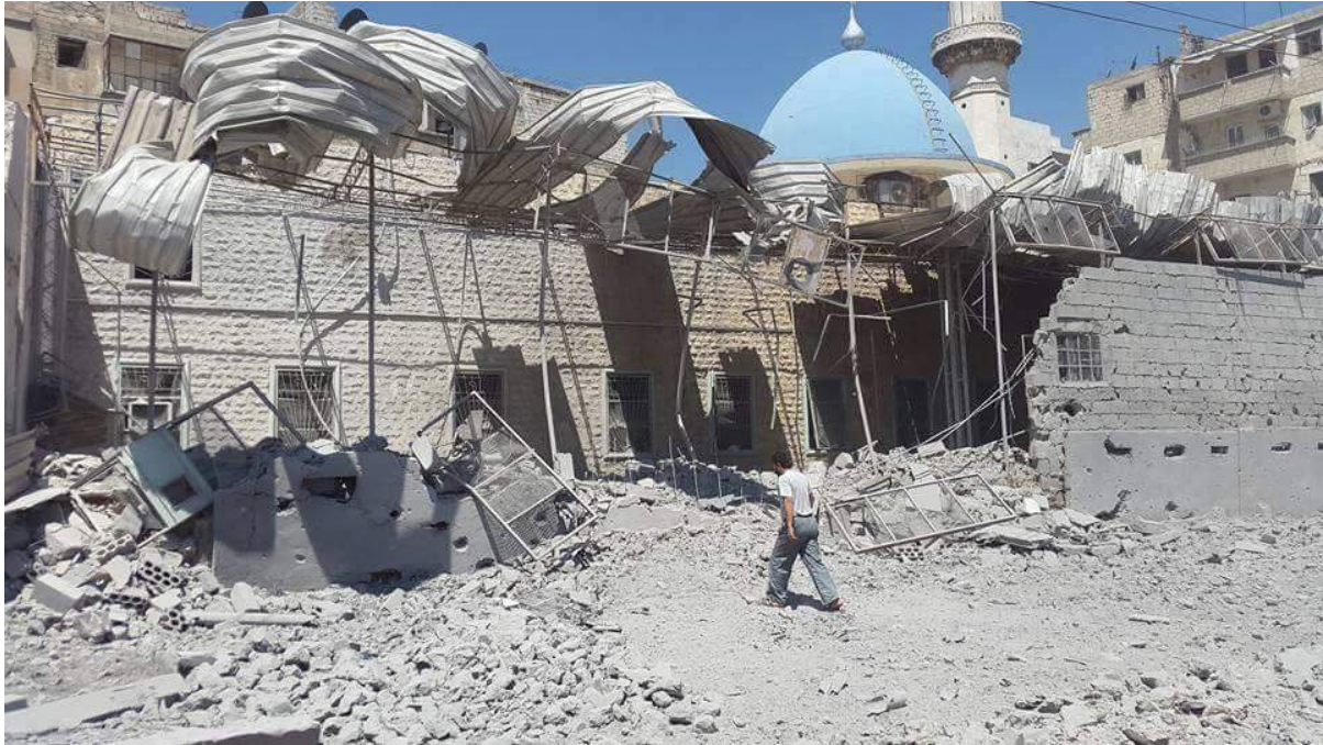
Damage to Oweis Al Karni Mosque (SNHR; April 29, 2016)
