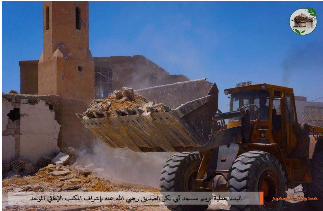
Removal of rubble from outside of the Abu Bakr al-Sidiq Mosque (Integrated Relief Office for Dumeir; May 6, 2016)
