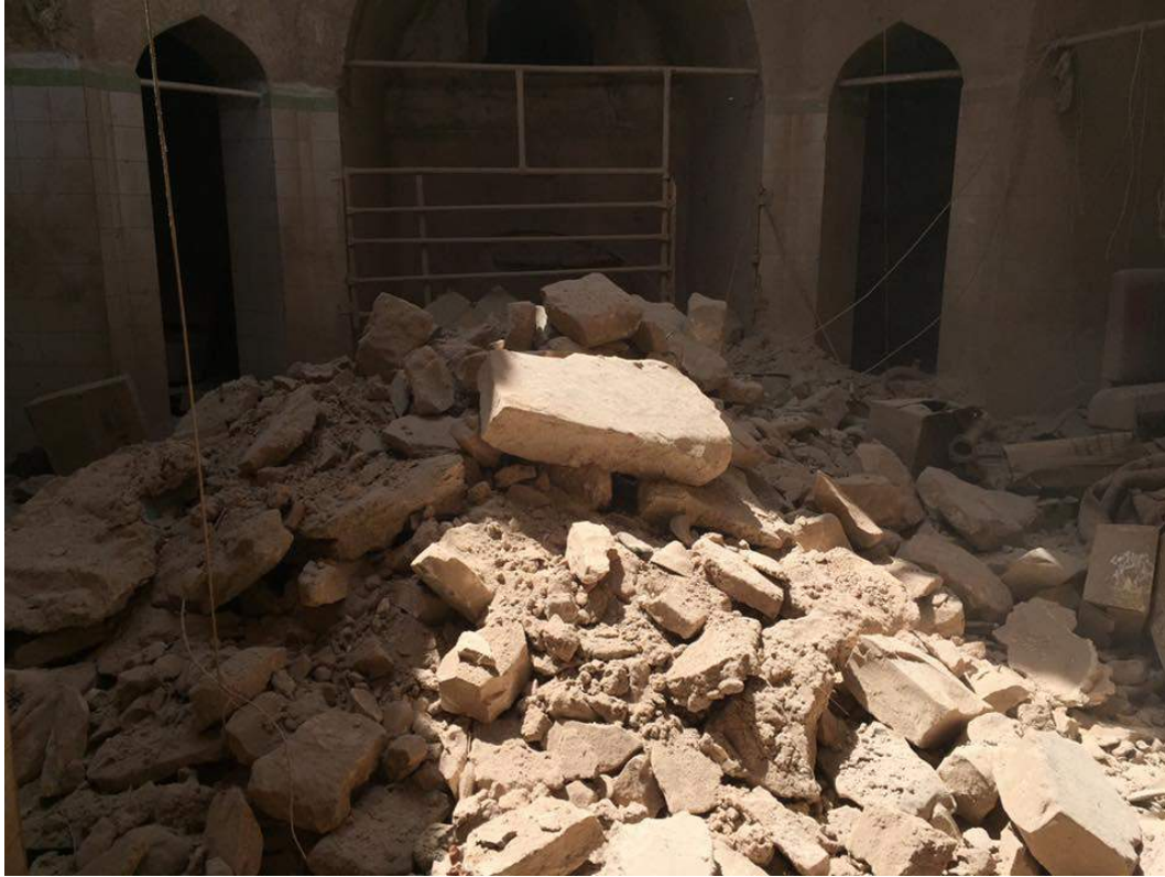
Interior damage at the Al-Ma'arra Museum (Al Watan FM; May 9, 2015)
