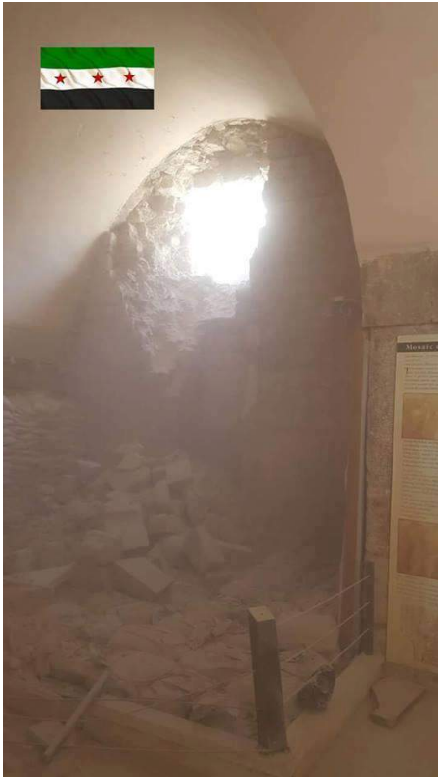
Airstrike damage at the Al-Ma'arra Museum (Republished by APSA; May 9, 2016)
