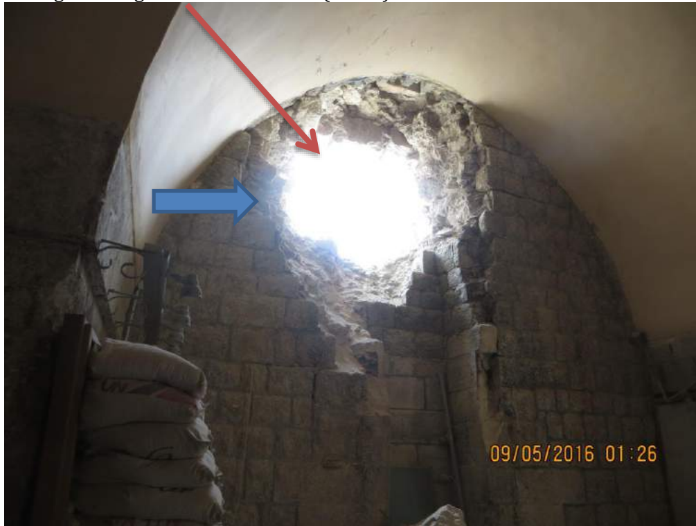
Damage causing a breach in the wall (inside)
