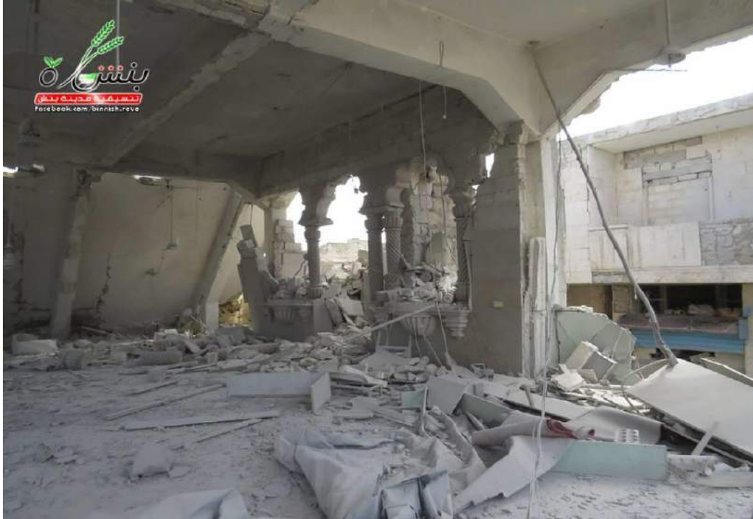
Interior damage to Sheikh Shuayab Mosque (Coordinators of the Revolution in the city of Binnish; May 10, 2016)
