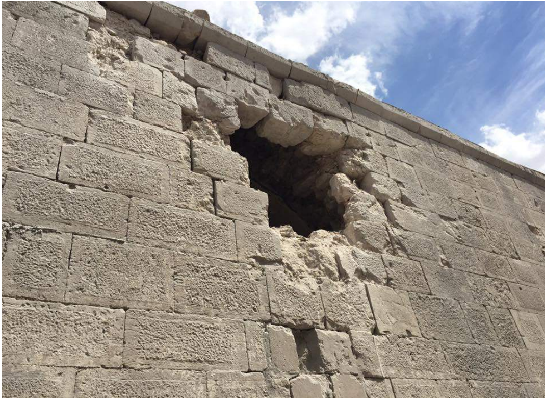
Damage to an exterior wall of the Al-Ma'arra Museum (Al Watan FM; May 9, 2015)
