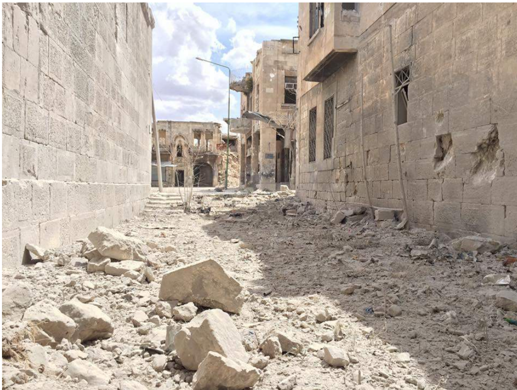
Damage to the exterior of the Al-Ma'arra Museum (Al Watan FM; May 9, 2015)
