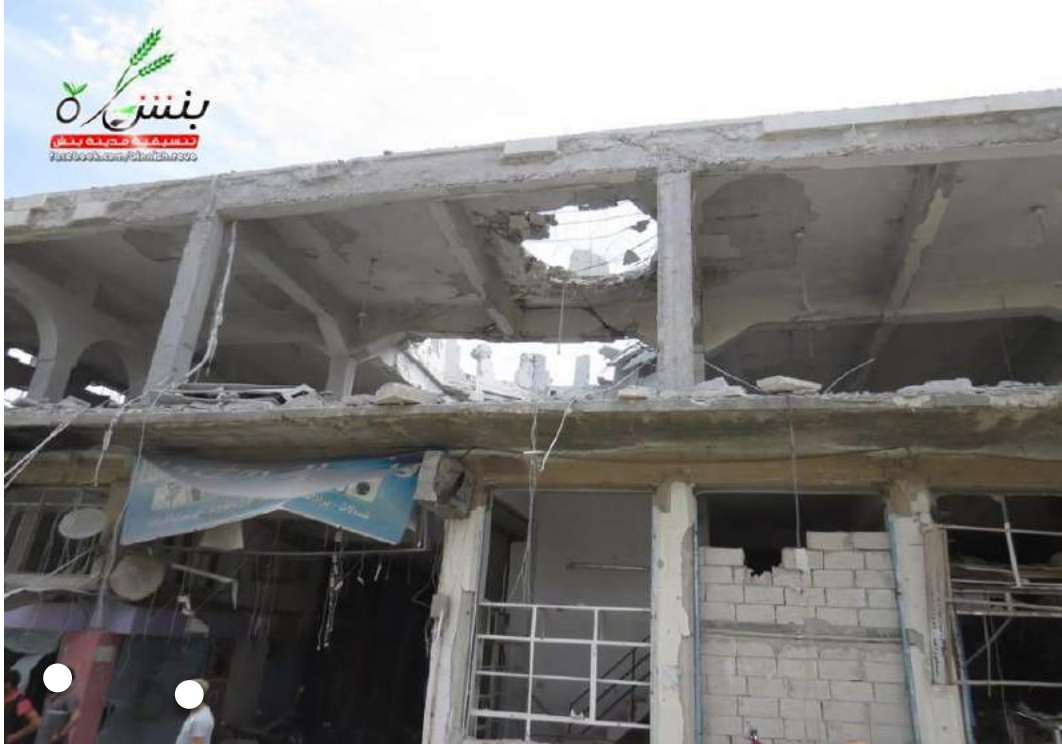
Photograph showing hole through the roof of Sheikh Shuayab Mosque (Coordinators of the Revolution in the city of Binnish; May 10, 2016)
