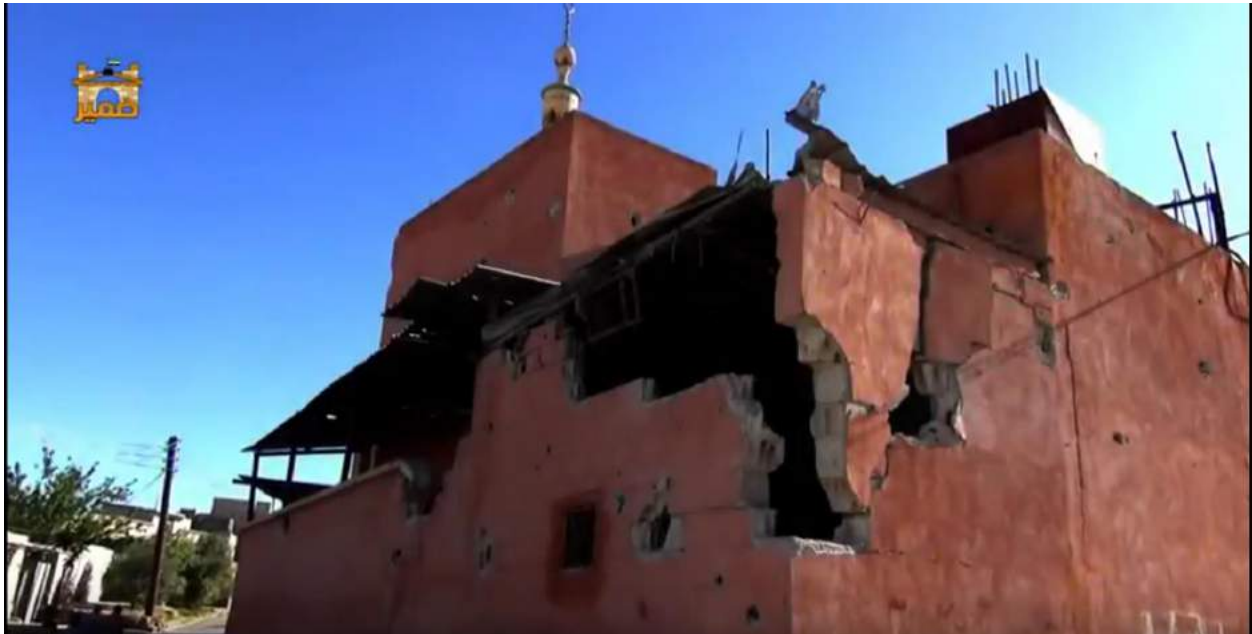
Damage to the exterior of the Abu Bakr al-Sidiq Mosque (Media Abu Mohammad; April 28, 2016)
