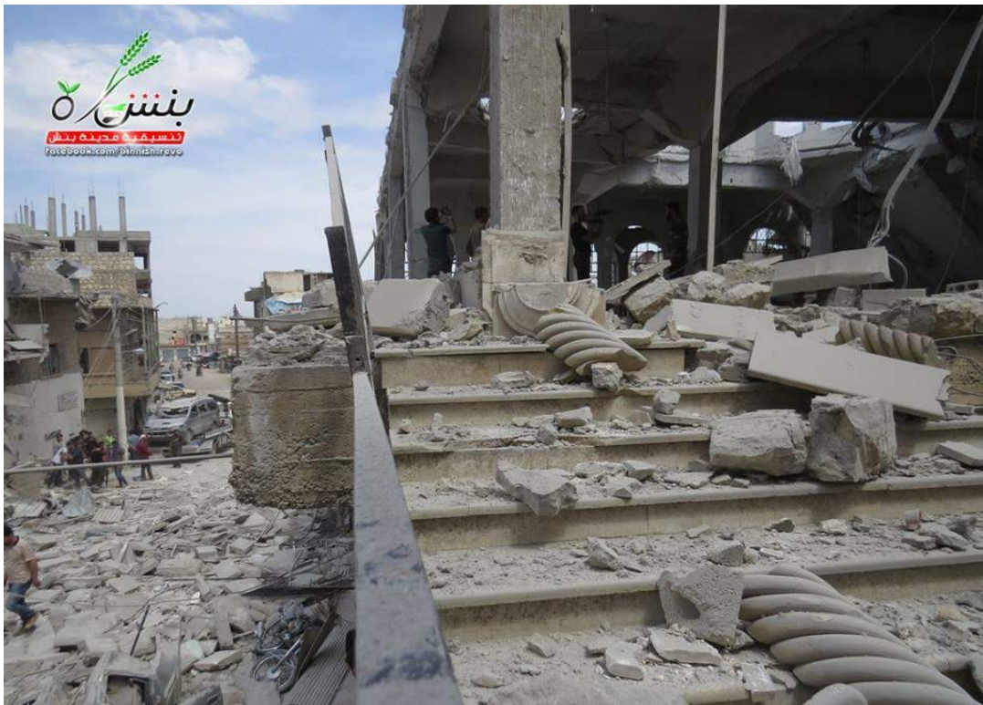
Exterior damage to the Sheikh Shuayab Mosque and nearby rubble on the street and stairs (Coordinators of the Revolution in the city of Binnish; May 10, 2016)
