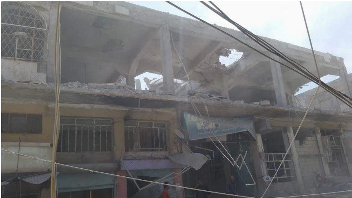
Photograph showing severe damage to Sheikh Shuayab Mosque (SNHR; May 10, 2016)
