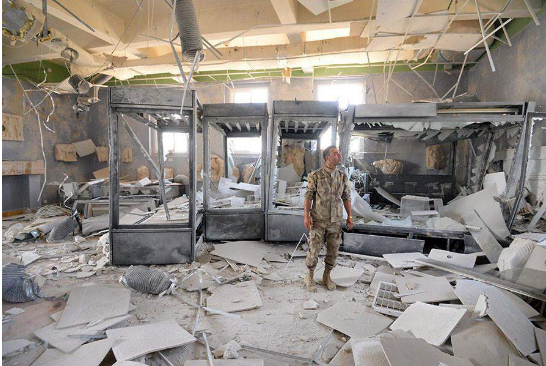
The damage to interior of Hall 3 of the Palmyra Museum (ABNA 24; March 28, 2016)
