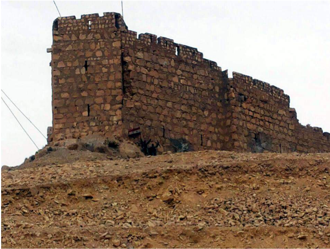
Minor airstrike damage to northwestern curtain wall (DGAM; March 26, 2016)
