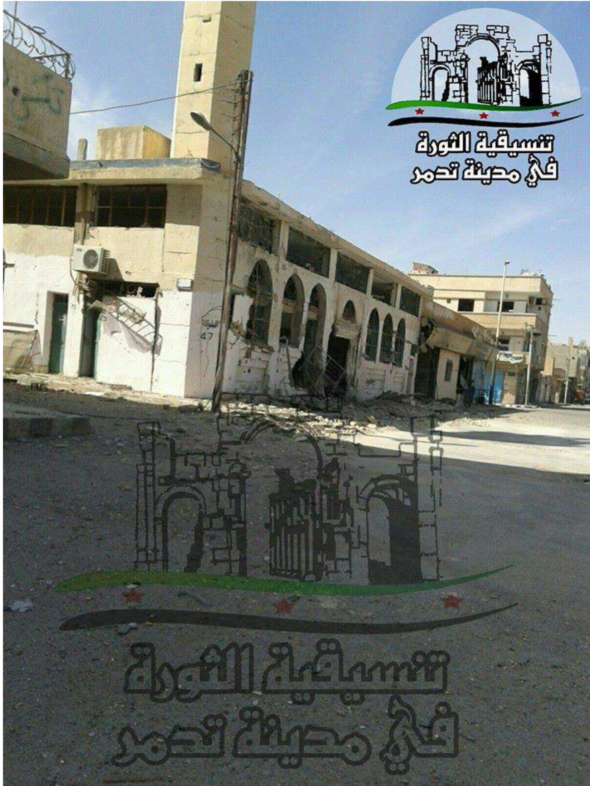
Damage to exterior of Bilal ibn Rabia Mosque (Palmyra Coordination; March 22, 2016)
