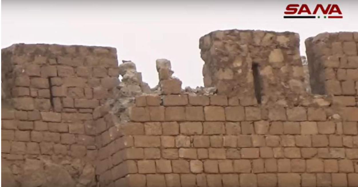
Partial collapse of eastern battlement (SANA; March 27, 2016)
