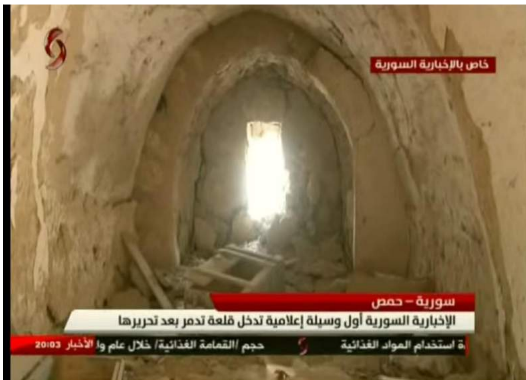
Debris and minor damage to interior of fortress and window (Syrian News Channel; March 26, 2016)
