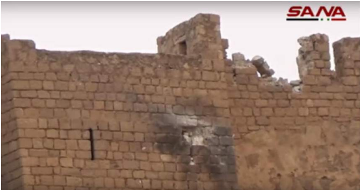
Airstrike damage to eastern curtain wall and partial collapse of battlement (SANA; March 27, 2016)
