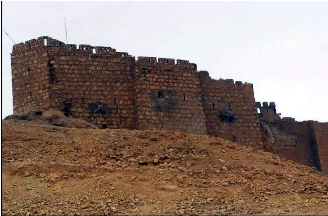
Airstrike damage to western walls (APSA; March 26, 2016)
