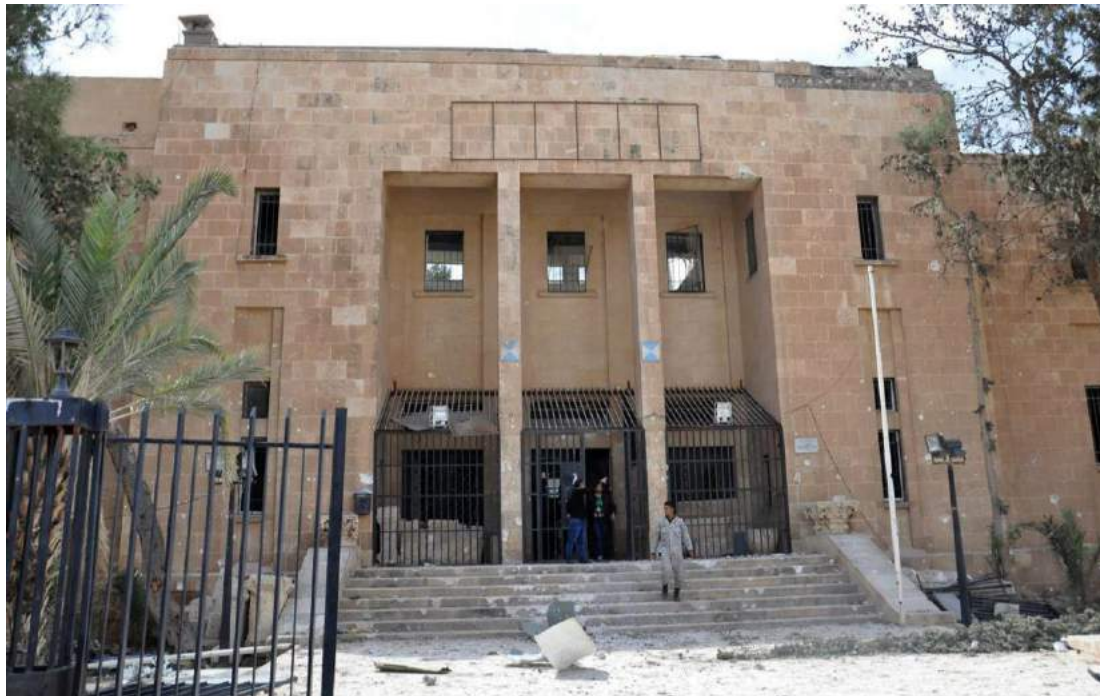
Damage to the exterior of the Palmyra Museum (SANA; March 29, 2016) 182
