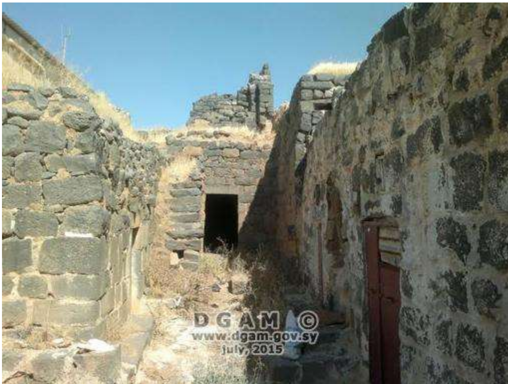
Old Houses, Marbaa, after destruction (DGAM; July 20, 2015)
