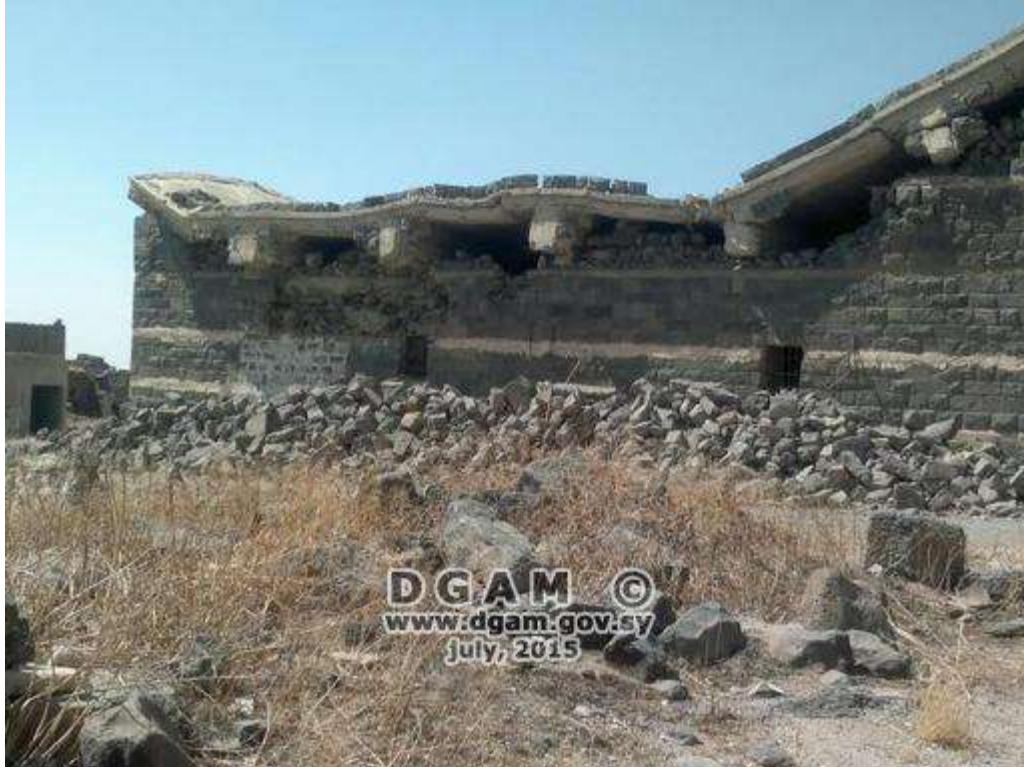
Al-Omari Mosque, Marbaa, after destruction (DGAM; July 15, 2015)
