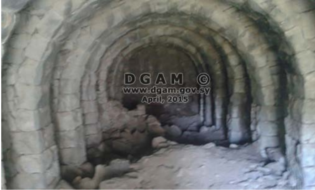
al-Khoubi house, Nawa, combat damage (DGAM; posted May 1, 2015)
