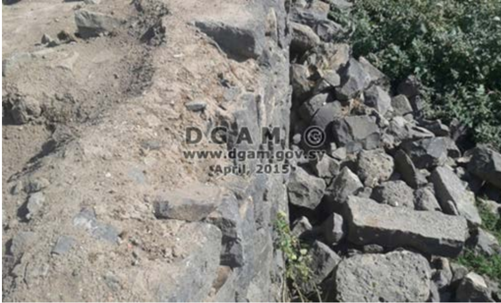
al-Jehmani house, Nawa, combat damage (DGAM; posted May 1, 2015)
