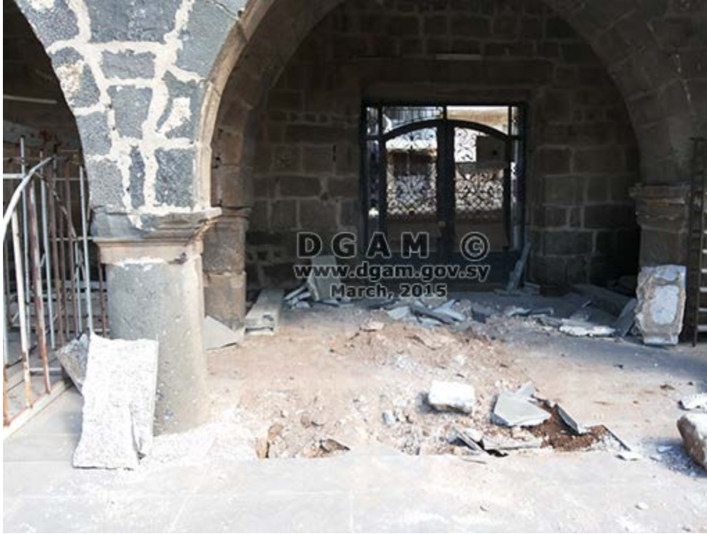
Omari Mosque, Daraa, Syria, showing digging inside the eastern door (DGAM; posted April 29, 2015)
