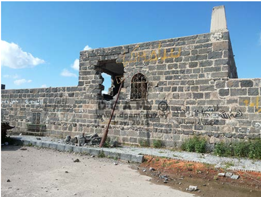
Omari Mosque, Daraa, Syria, showing damage to the south facade (DGAM; posted April 29, 2015)
