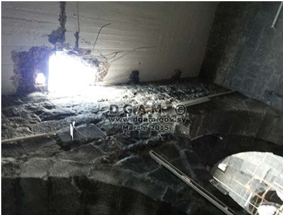
Omari Mosque, Daraa, Syria, showing damage to the roof to the left of the mihrab (DGAM; posted April 29, 2015)
