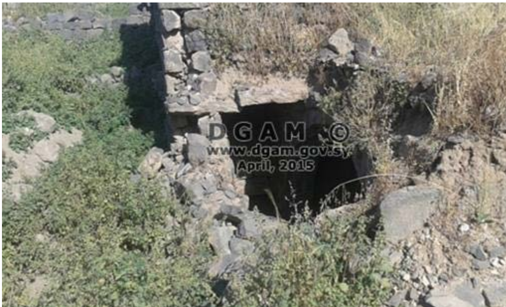
al-Batha house, Nawa, combat damage (DGAM; posted May 1, 2015)
