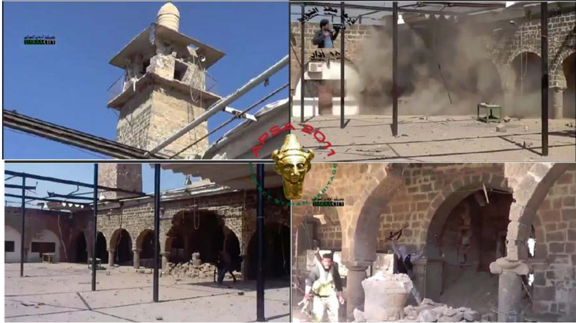
Omari Mosque, Daraa, Syria (APSA, Facebook page; posted March 22 2013). Images showing the condition of the courtyard and minaret due to prolonged siege and combat damage.
