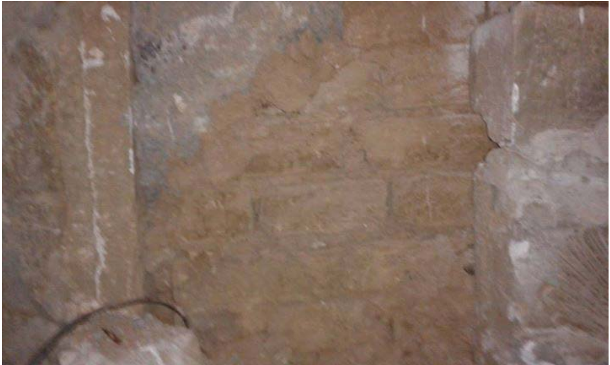
Alleged damage to the Northwest Palace at Nimrud, dating to October 2014 (Facebook)
