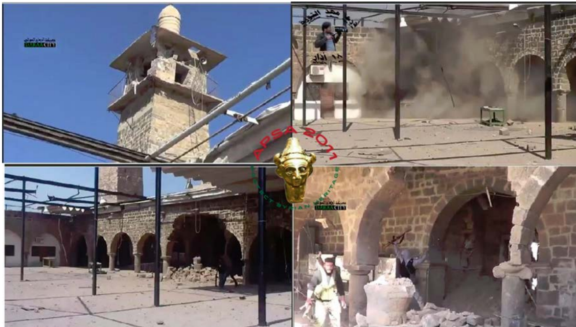
Omari Mosque, Daraa, Syria. Images showing the condition of the courtyard and minaret due to prolonged siege and combat damage. (APSA, Facebook page; posted March 22 2013)
