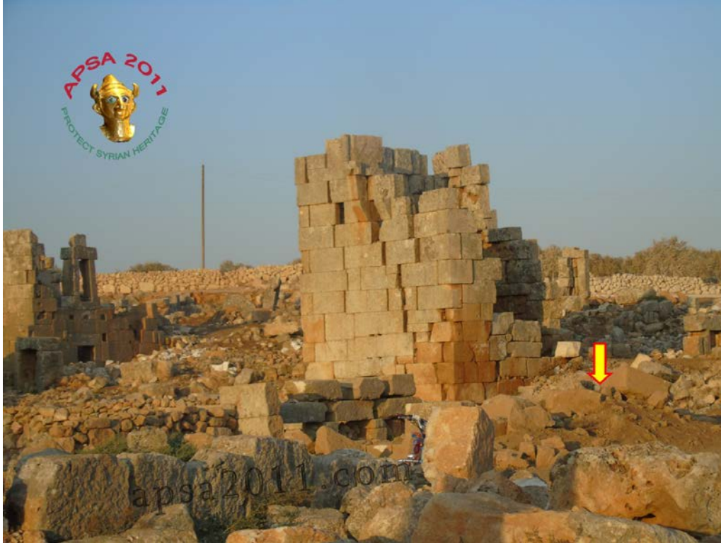
Deir Qita — an area of heavy disturbance at on the right possibly marking looting. (APSA)
