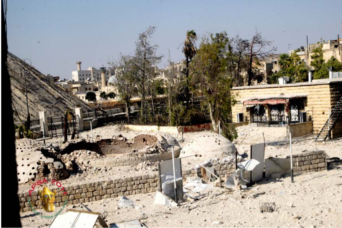
Damage to one of the domes of the Hammam Yalbougha (bathhouse) in Old Aleppo (APSA).
