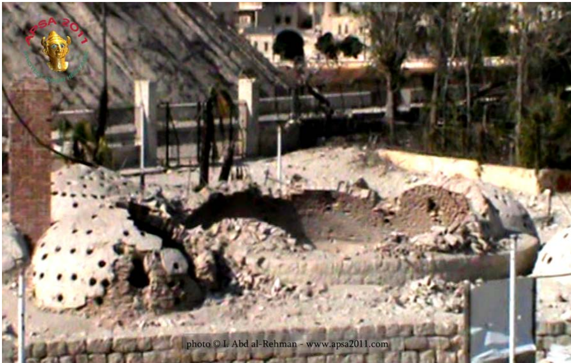
Damage to one of the domes of the Hammam Yalbougha (bathhouse) in Old Aleppo (APSA).
