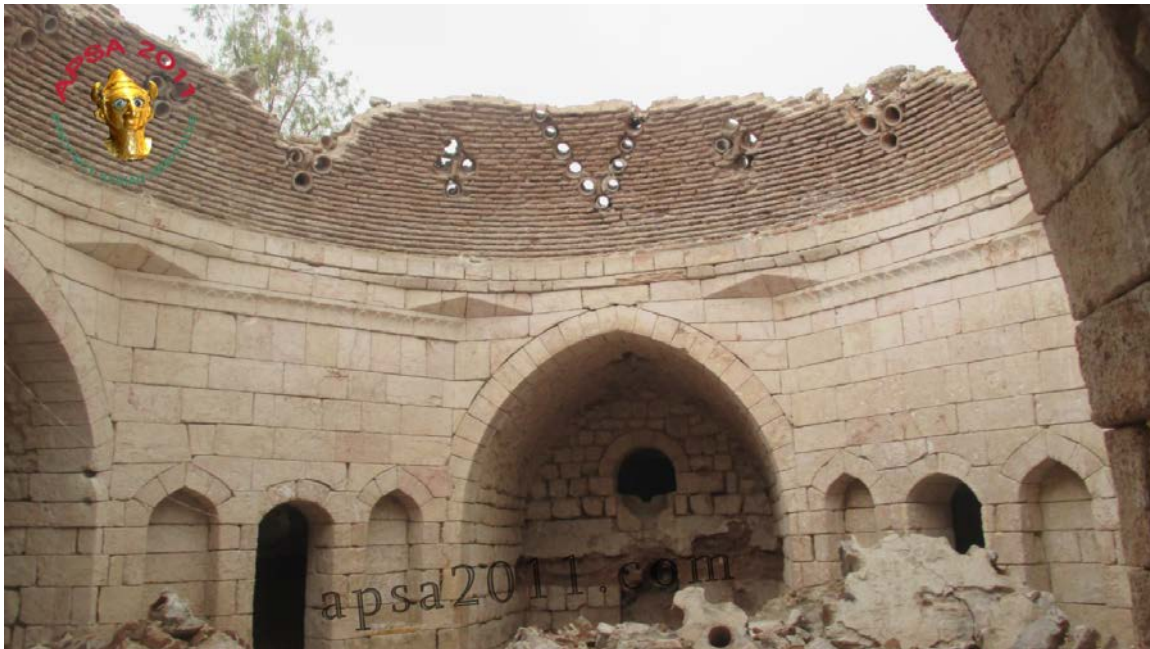
Damage to one of the domes of the Hammam Yalbougha (bathhouse) in Old Aleppo (APSA).
