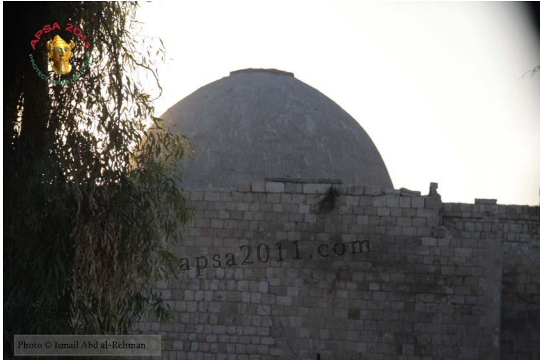
Damage to one of the domes of the Hammam Yalbougha (bathhouse) in Old Aleppo (APSA).
