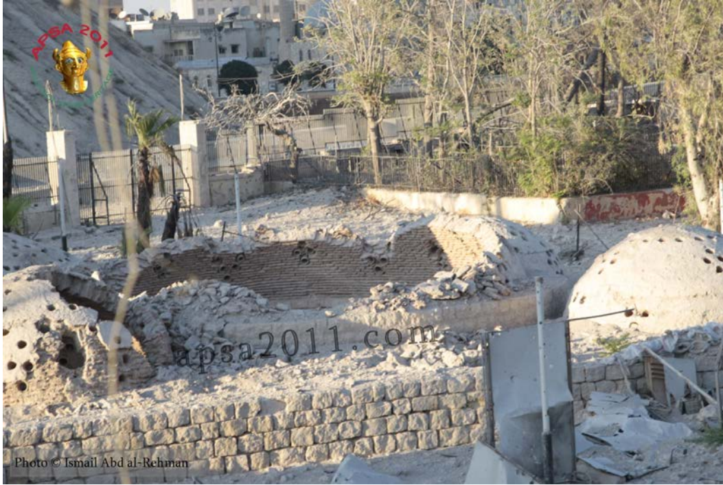
Damage to one of the domes of the Hammam Yalbougha (bathhouse) in Old Aleppo (APSA).
