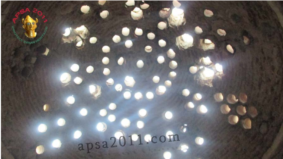
Damage to one of the domes of the Hammam Yalbougha (bathhouse) in Old Aleppo (APSA).
