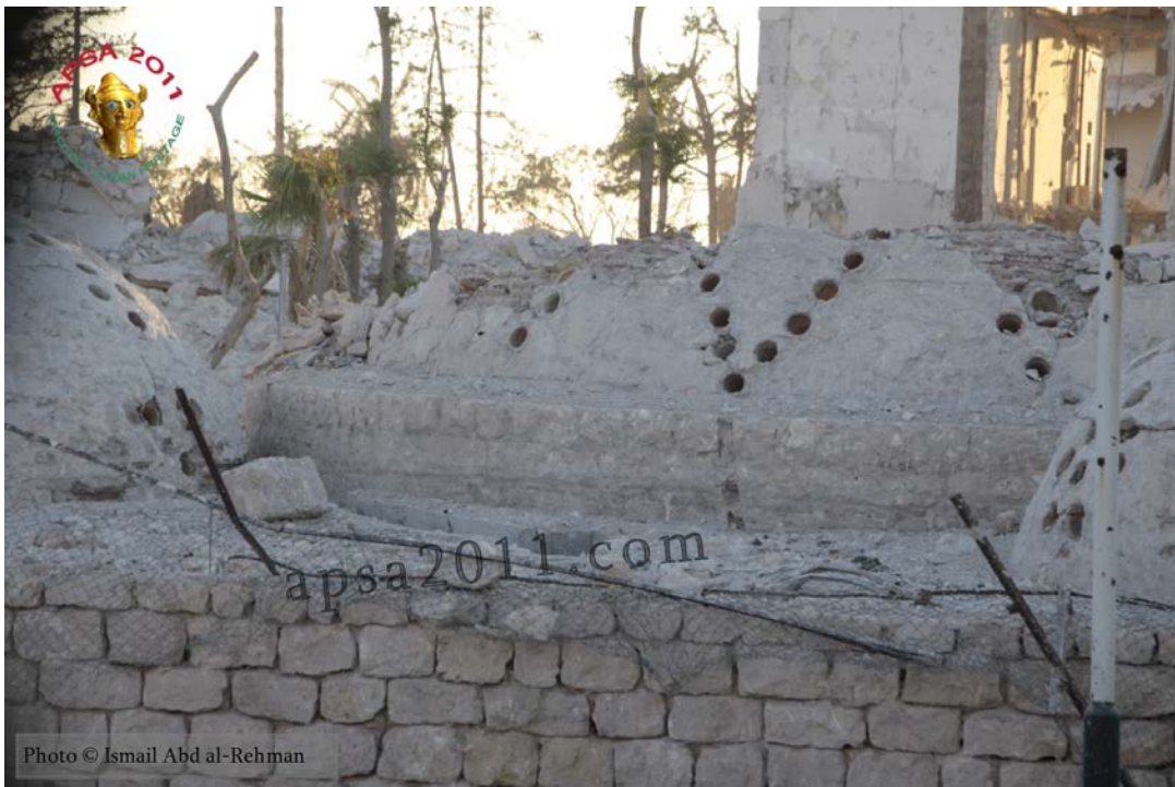
Damage to one of the domes of the Hammam Yalbougha (bathhouse) in Old Aleppo (APSA).
