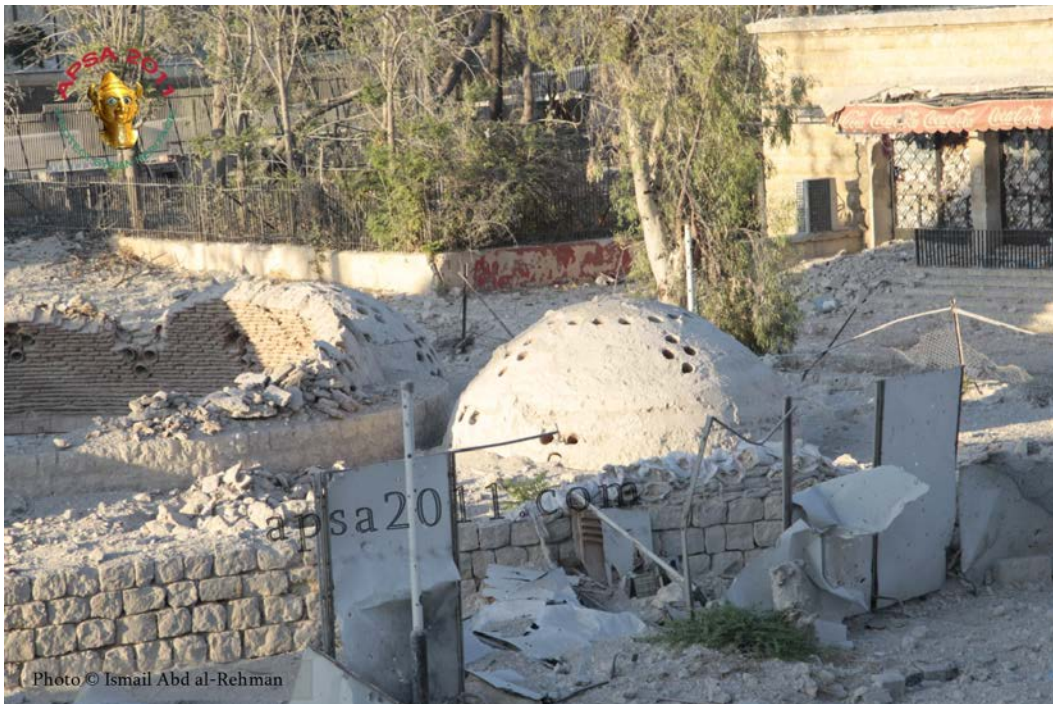
Damage to one of the domes of the Hammam Yalbougha (bathhouse) in Old Aleppo (APSA).
