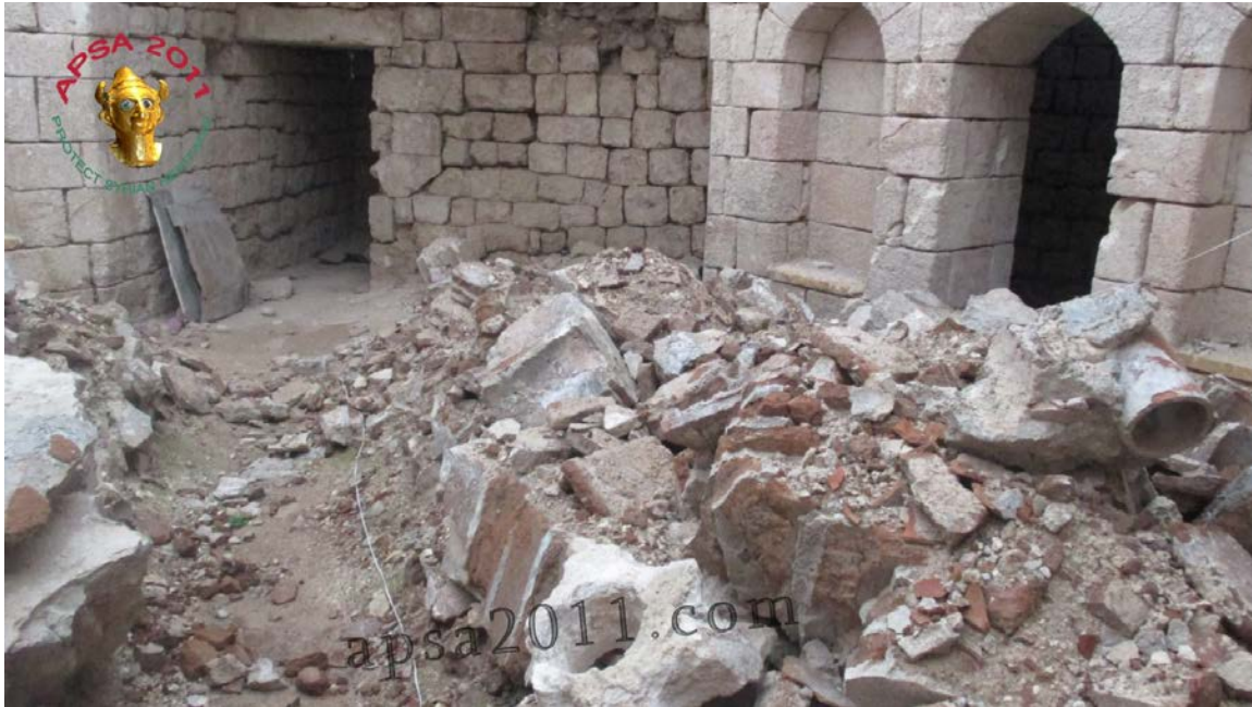
Damage to the Hammam Yalbougha (bathhouse) in Old Aleppo (APSA).
