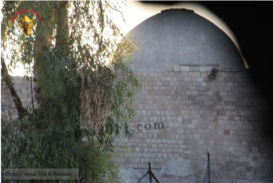
Damage to one of the domes of the Hammam Yalbougha (bathhouse) in Old Aleppo (APSA).
