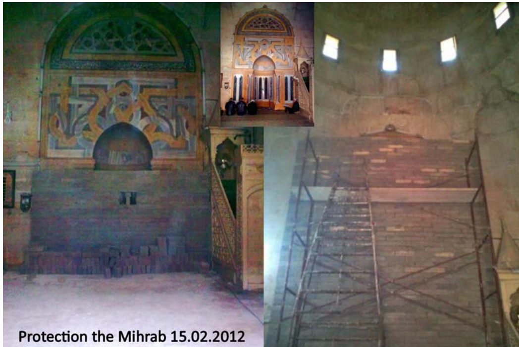
Protection the Mihrab 15.02.2012 Mihrab of the Madrasa Firdows in Aleppo (APSA).
