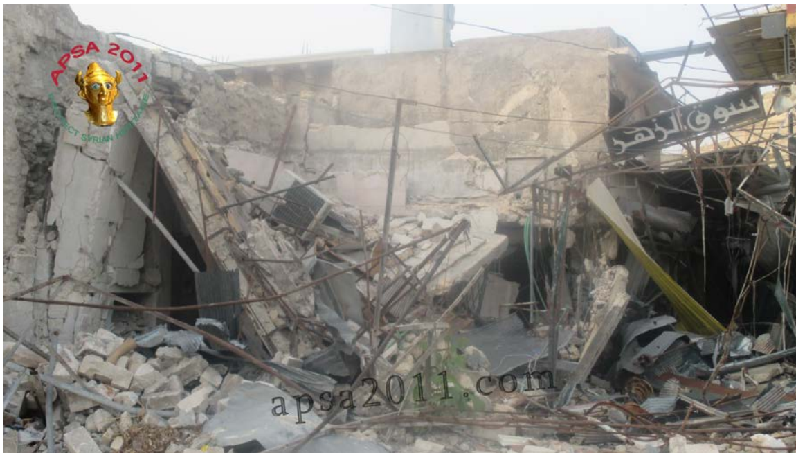
Recent photo of damage in the Suq Bab al-Hadid (APSA).
