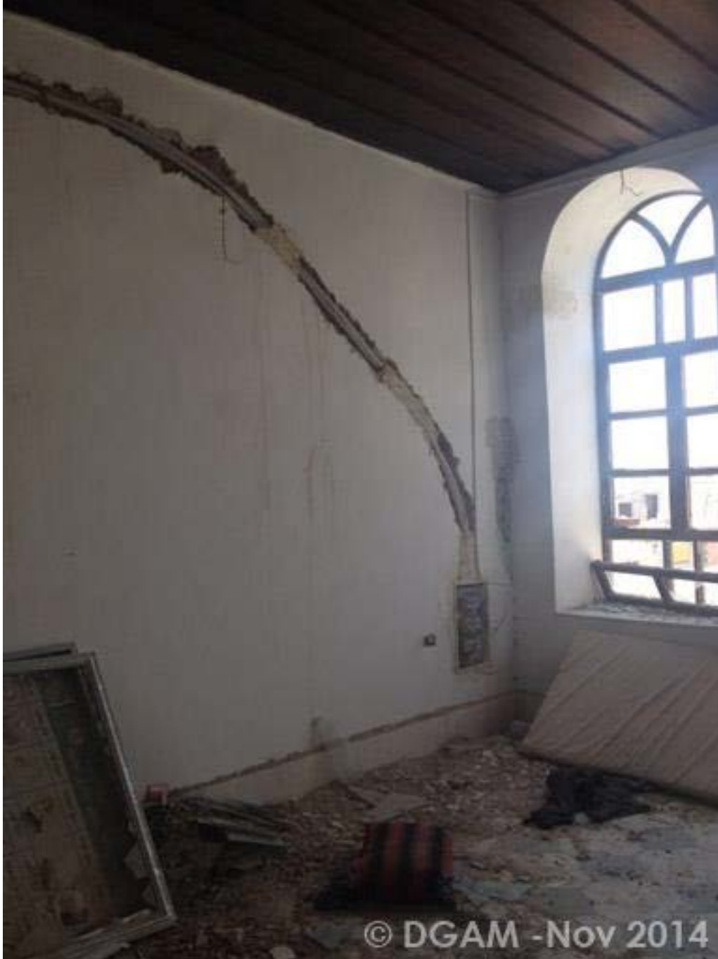
Damage to the Seray Building in Al-Nabk (DGAM).
