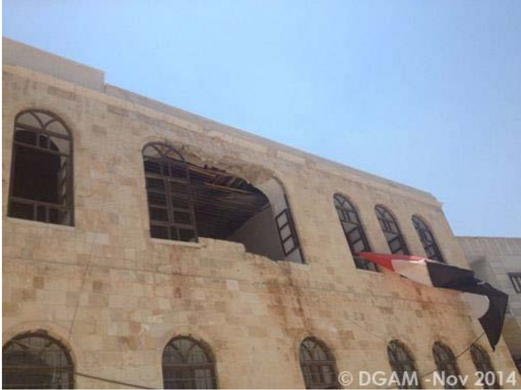
Damage to the Seray Building in Al-Nabk (DGAM).
