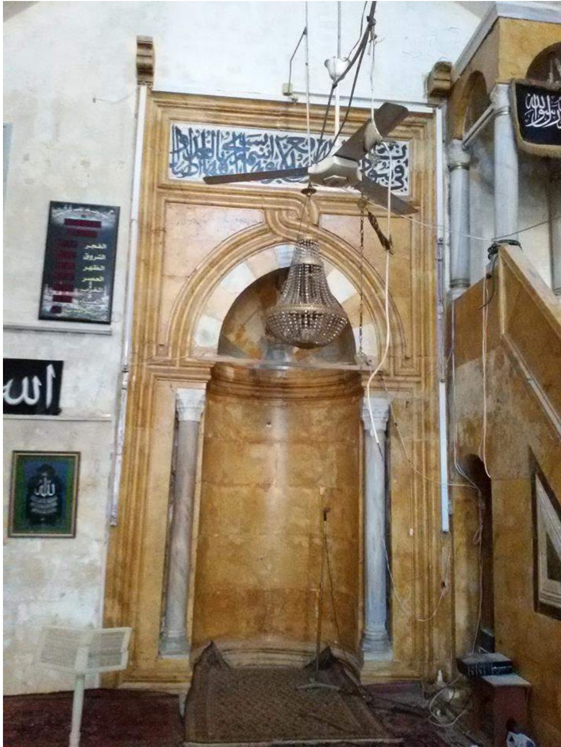
Slight damage to mihrab and minbar inside al-Sarawi Mosque (Private Facebook Account; December 10, 2016)
