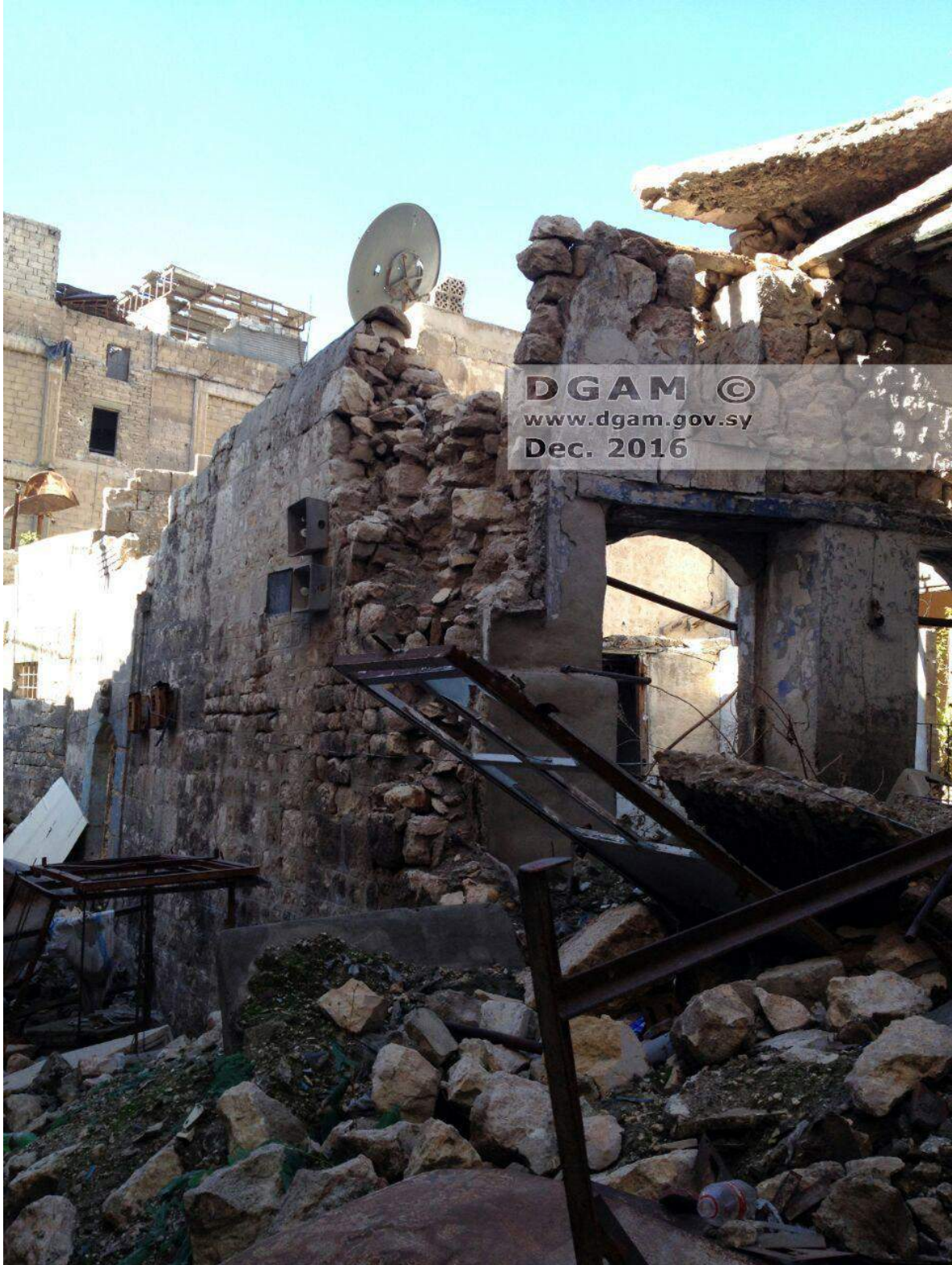
Severe damage to the Khan al-Harir building (DGAM; December 12, 2016)
