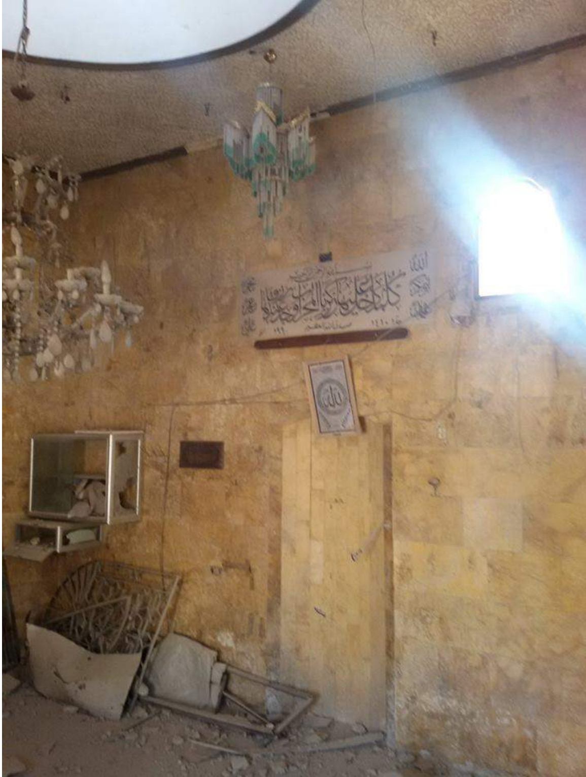
Rubble filled interior of al-Mesla Mosque (Private Facebook Account; December 10, 2016)
