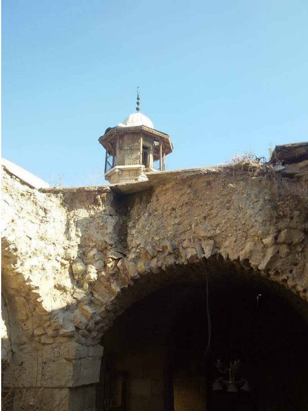
The minaret of al-Hadadeen Mosque is seen above the heavily damaged mosque (Private Facebook Account; December 10, 2016)
