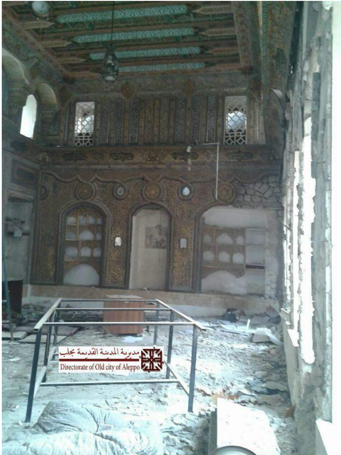
Damage to the interior of Dar Qatar Agassi (Rami M Alafandi; December 12, 2016)
