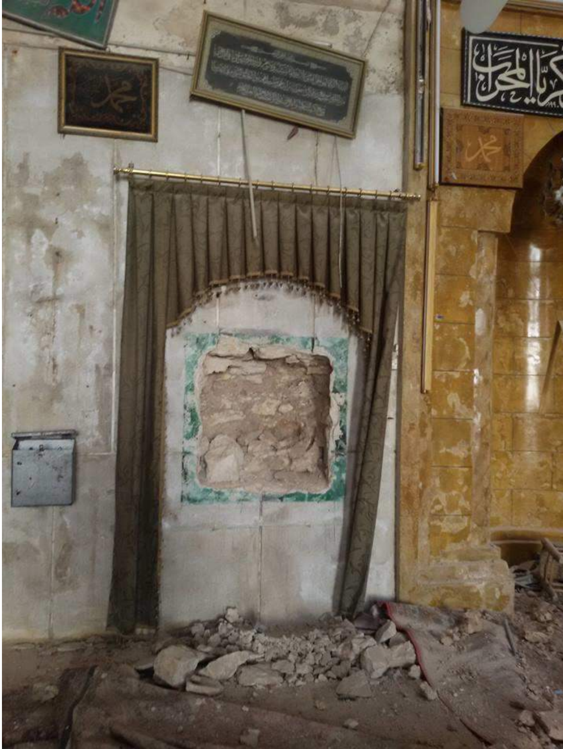
A photograph showing vandalism and theft of an unknown object at Banqusa Mosque (Private Facebook Account; December 10, 2016)
