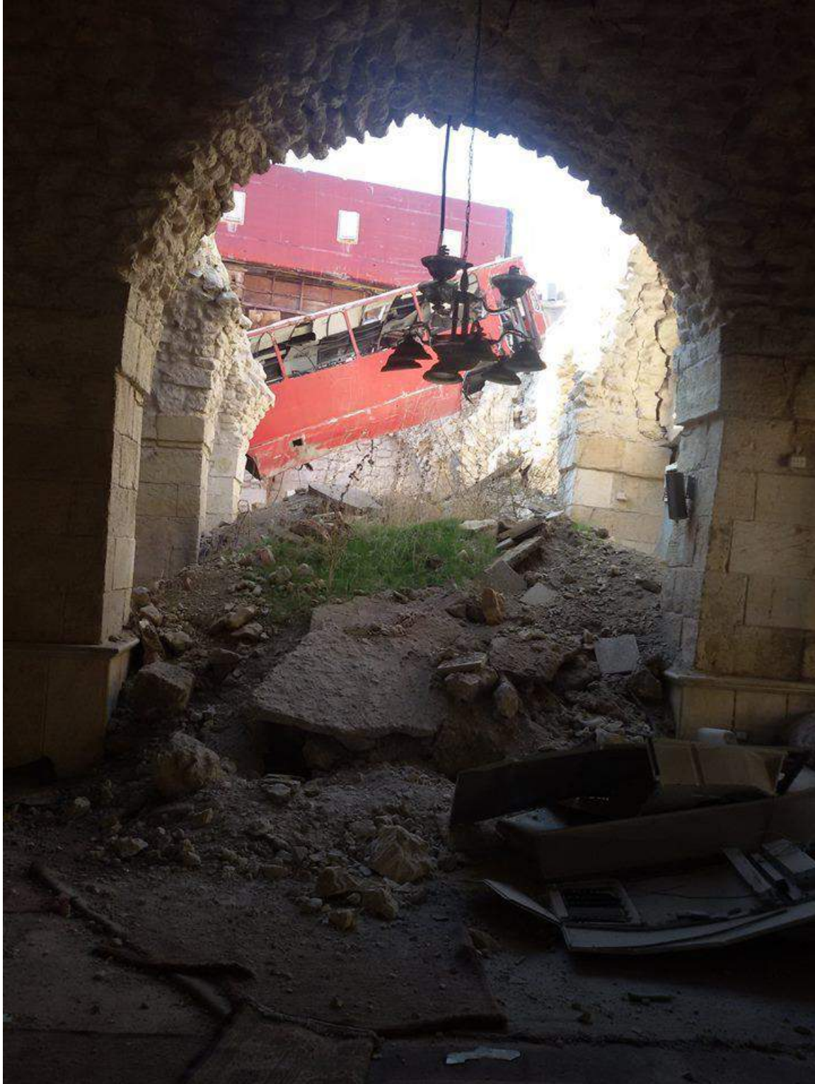
Severe structural damage to al-Hadadeen Mosque (Private Facebook Account; December 10, 2016)
