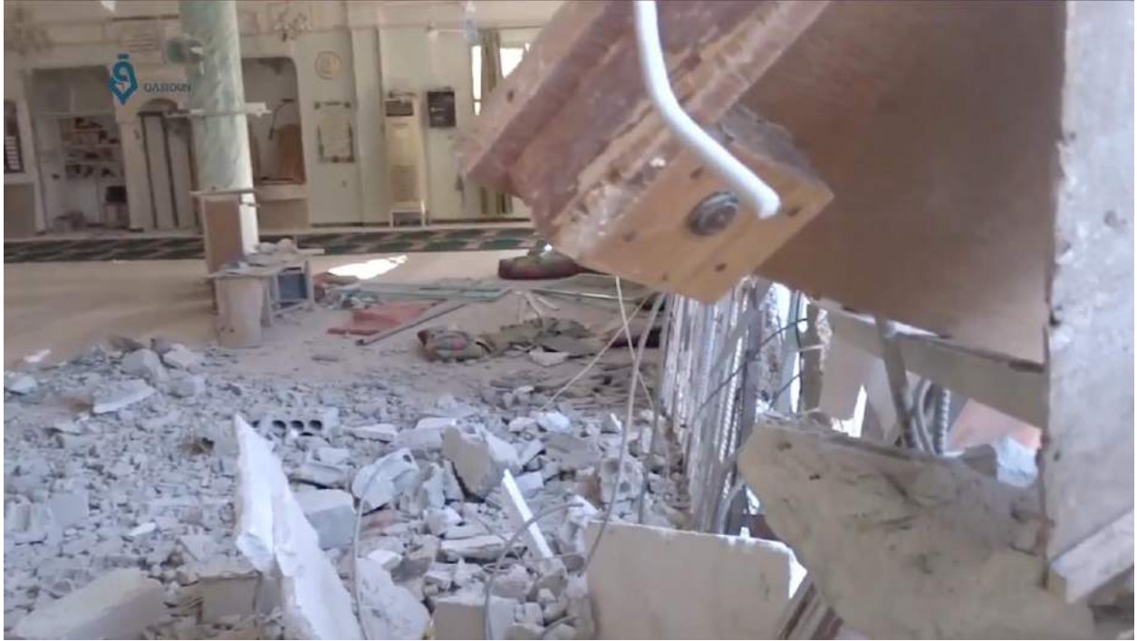
Video still shows damage to Omar bin al-Khattab Mosque (Qasioun News Agency; December 4, 2016)
