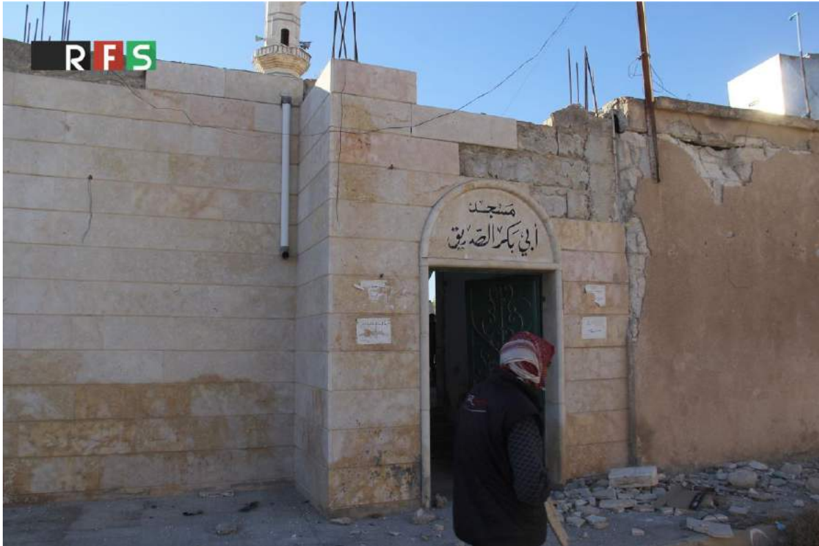
Damage to the exterior of Abu Bakr al-Sidiq Mosque (RFS Media; December 6, 2016)
