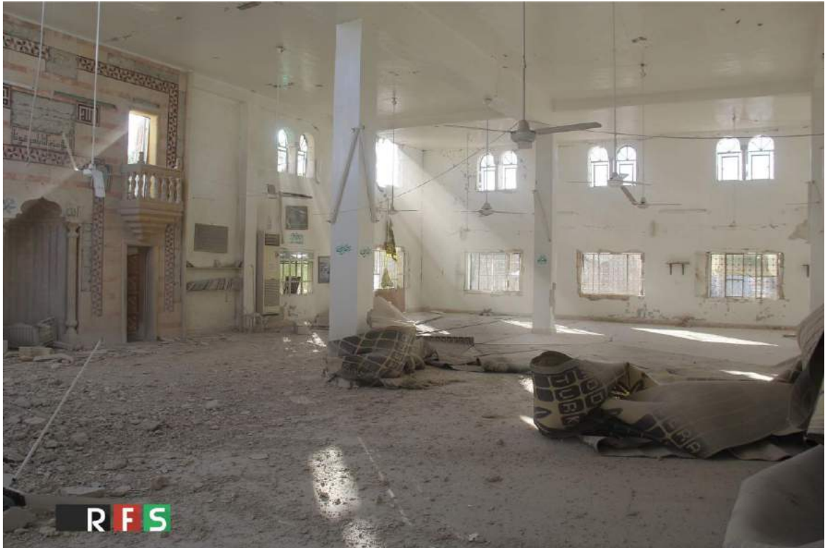
Damage to the interior of Abu Bakr al-Sidiq Mosque (RFS Media; December 6, 2016)
