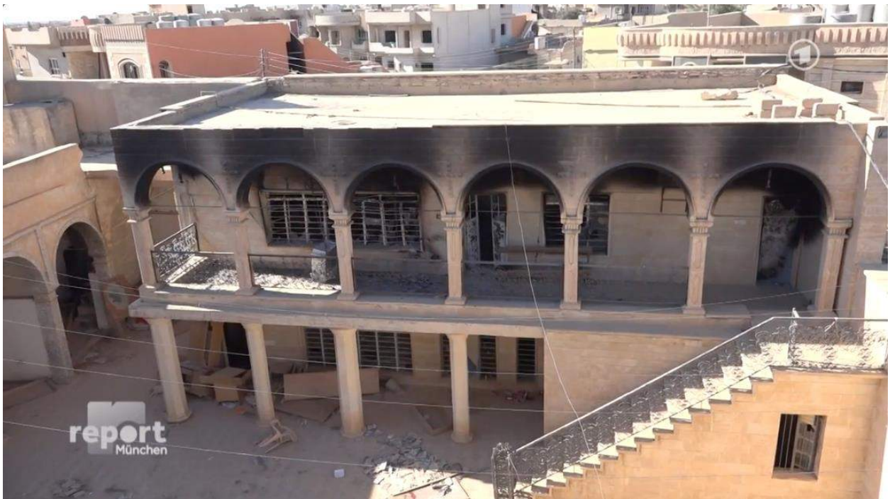
Video still of damage to the courtyard and building of Mart Shmone Church, fire damage apparent (Report München; December 7, 2016)
