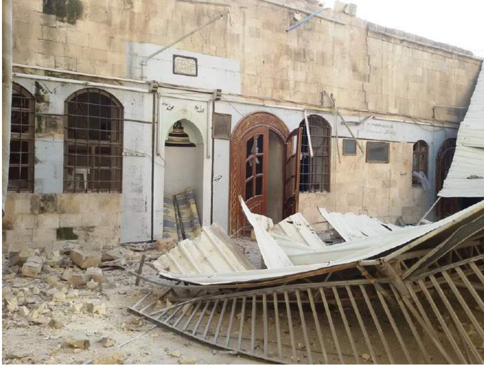
Moderate damage to the Qarleq Mosque, showing damaged roof (Private Facebook Account; December 10, 2016)
