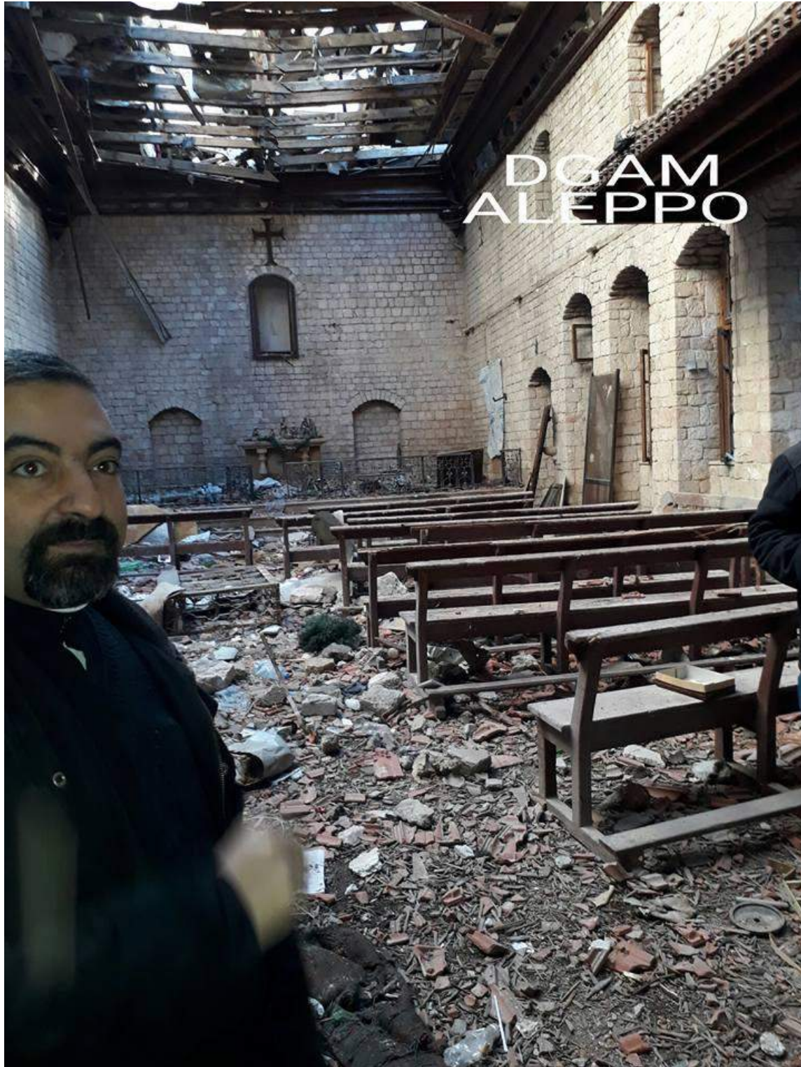
Damage to the interior of the Church of Our Lady (DGAM Aleppo; December 8, 2016)
