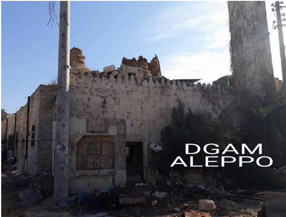
A heavily damaged Qastal al-Harami Mosque, likely with dome missing (DGAM Aleppo; December 8, 2016)
