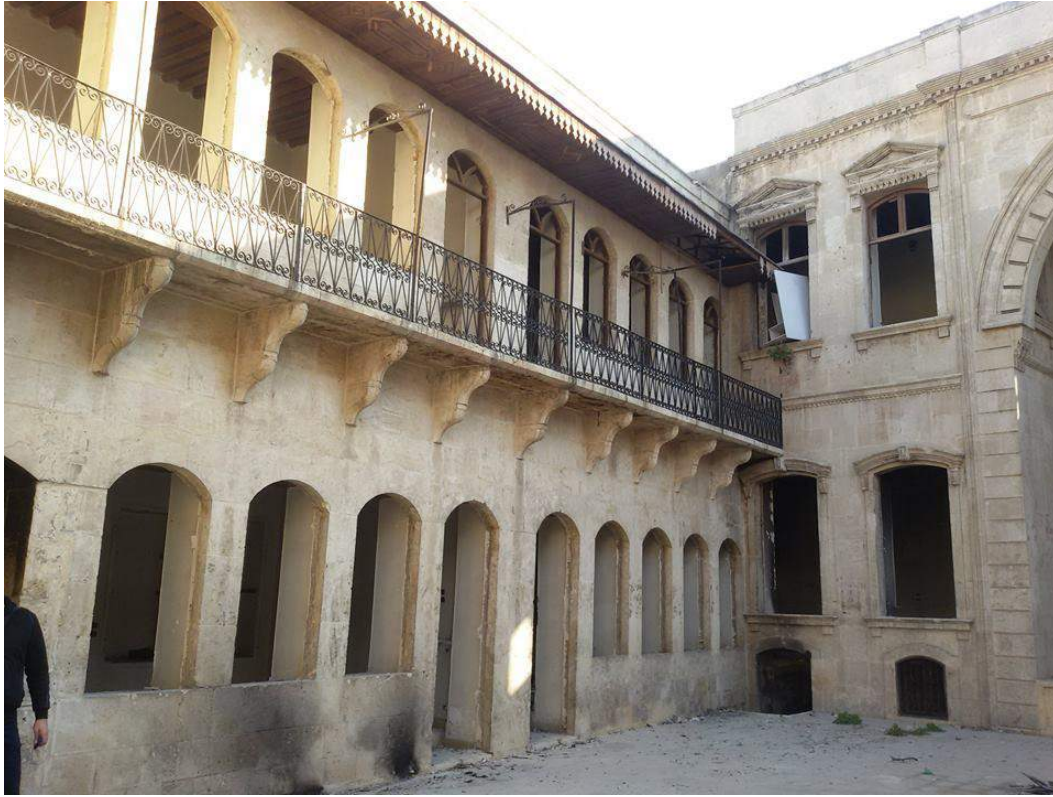
Minor damage to the Musa bin Nasir Madrassa showing missing windows, fire damage, and shrapnel holes (Private Facebook Account; December 10, 2016)
