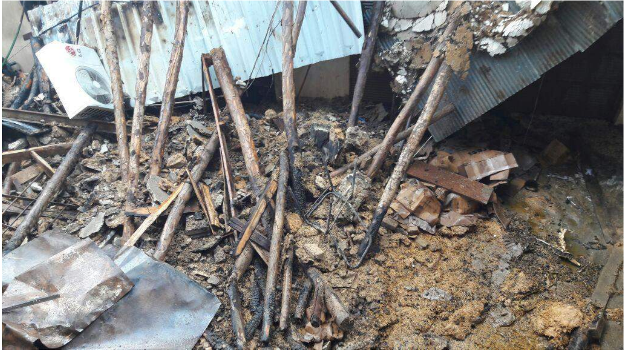
Fire damage in al-Hamidiyah Souq (DGAM; December 2, 2016)
