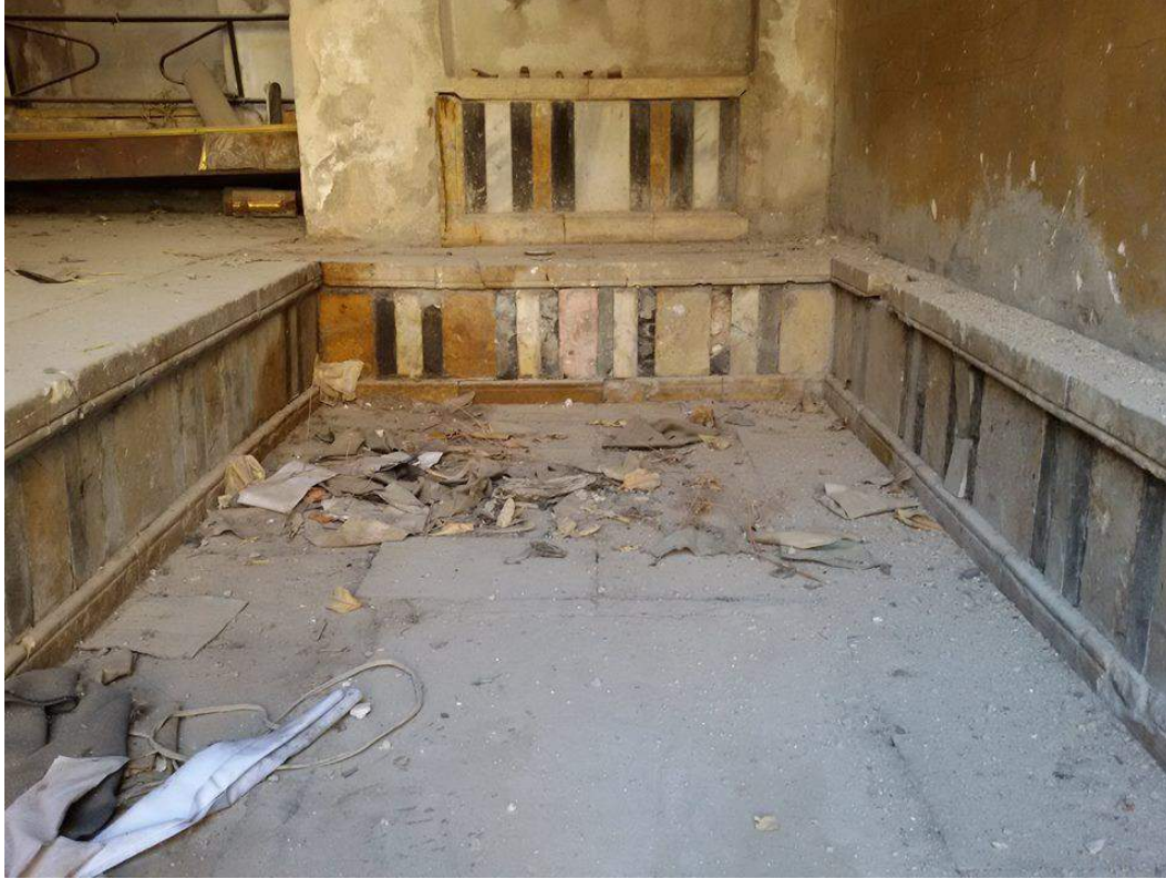
Slight damage to the courtyard or inside of the Old Arab House (Private Facebook Account; December 10, 2016)
