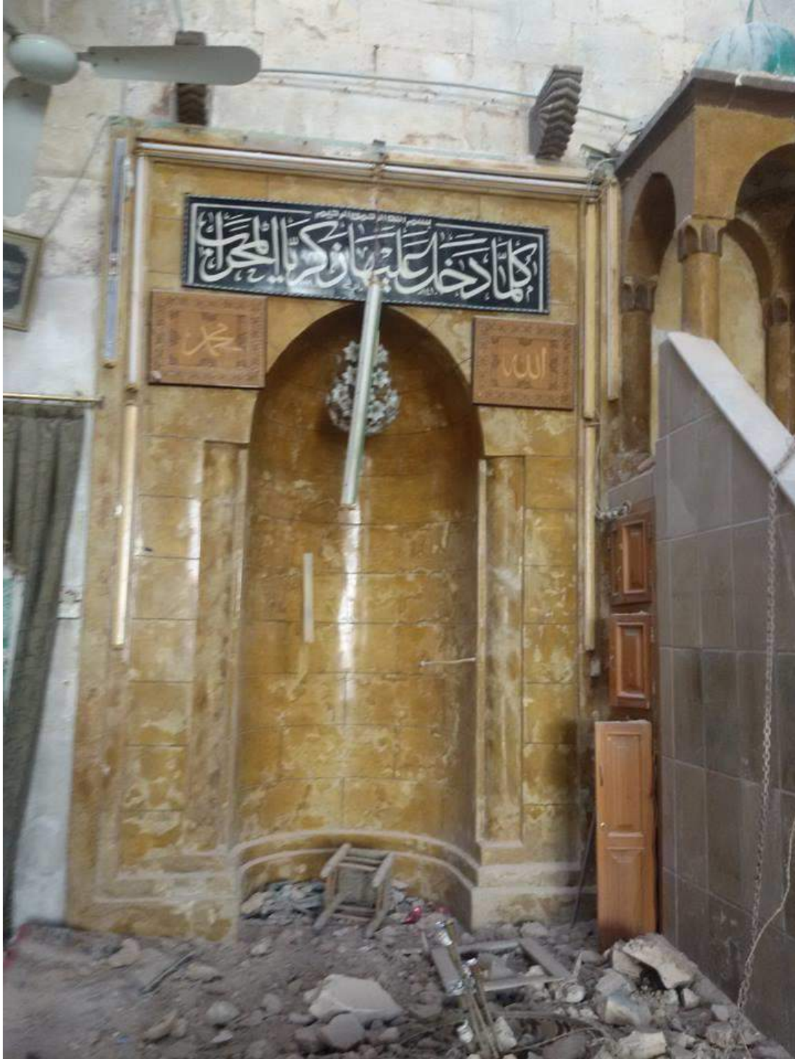
Detail of damage to the mihrab inside Banqusa Mosque (Private Facebook Account; December 10, 2016)
