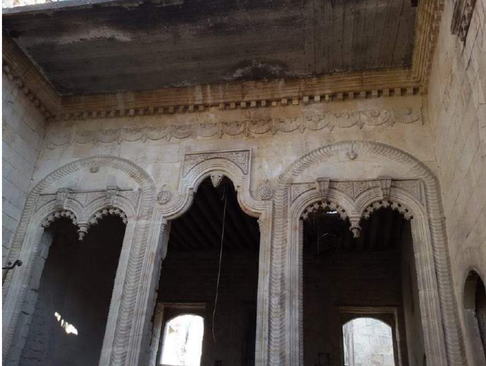
Moderate damage to inside of al-Sarawi Mosque showing fire damage (Private Facebook Account; December 10, 2016)
