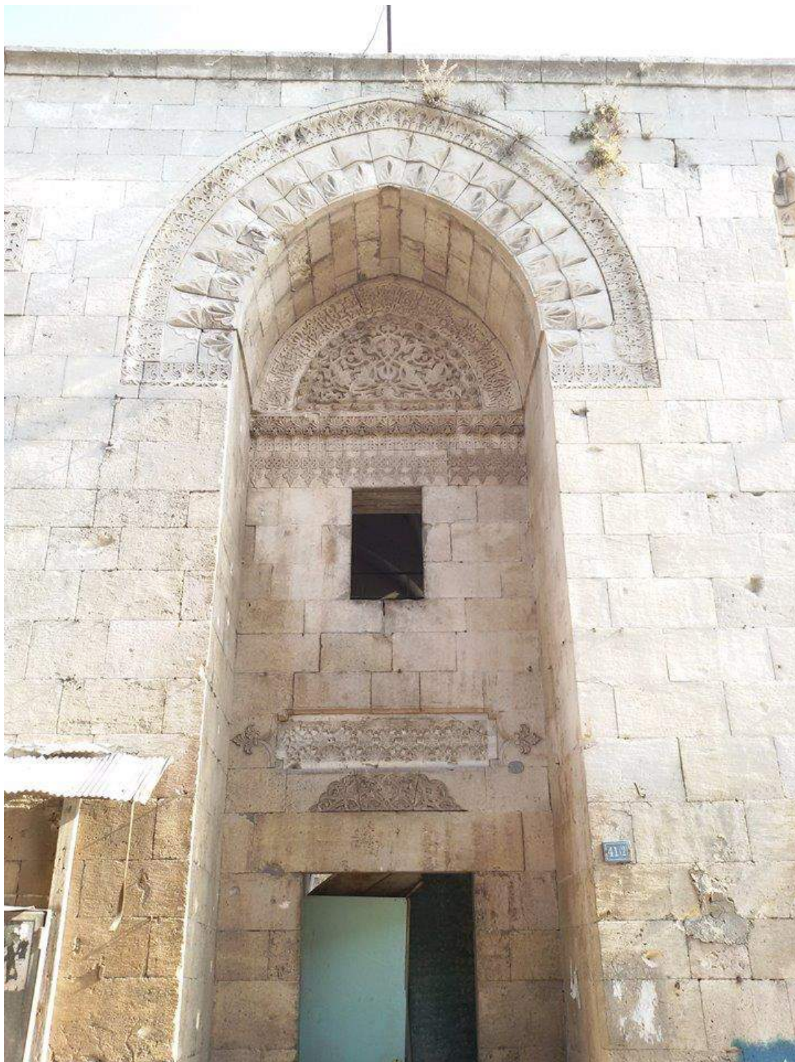
Light damage to al-Sarawi Mosque and Madrasa Muqabilat (Private Facebook Account; December 10, 2016)
