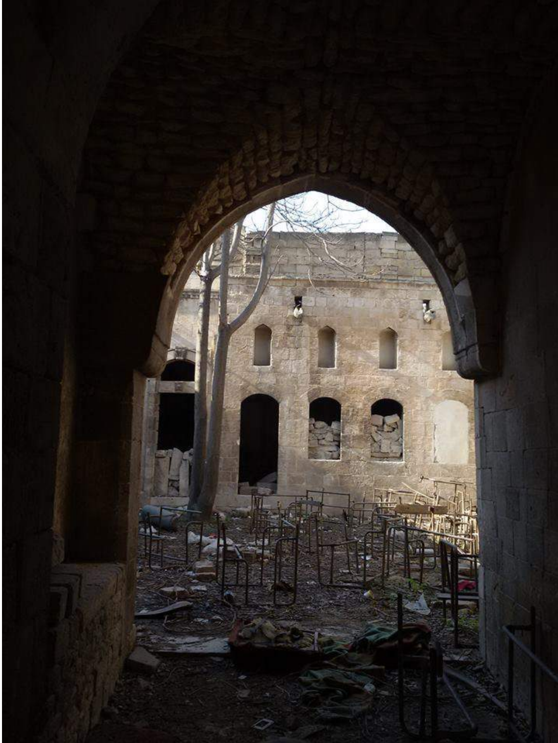
Damage in the courtyard of al-Sarawi Mosque and Madrasa Muqabilat (Private Facebook Account; December 10, 2016)
