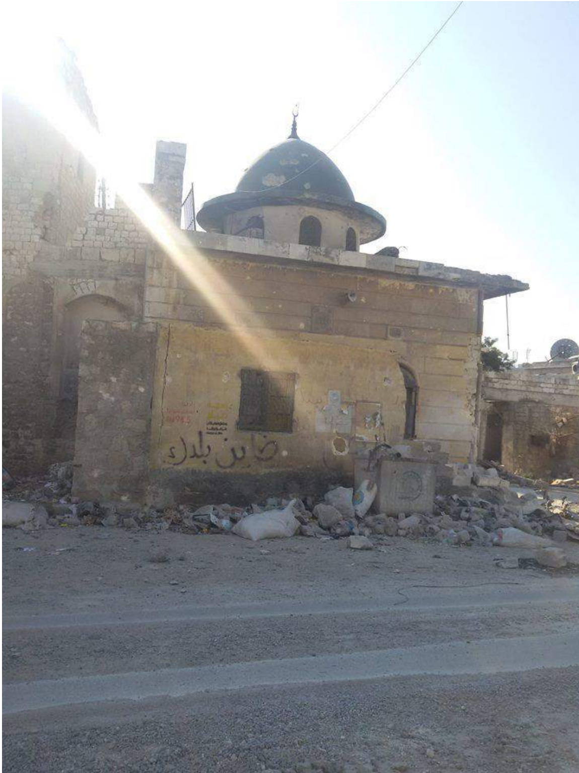
Moderate to severe damage to outside of al-Mesla Mosque (Private Facebook Account; December 10, 2016)
