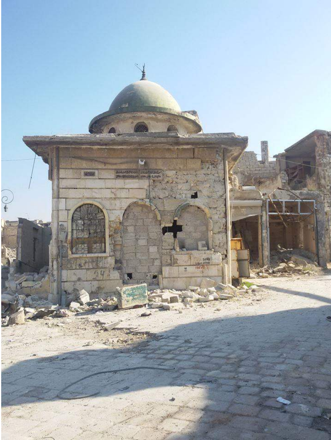
Moderate to severe damage to the outside of al-Mesla Mosque (Private Facebook Account; December 10, 2016)
