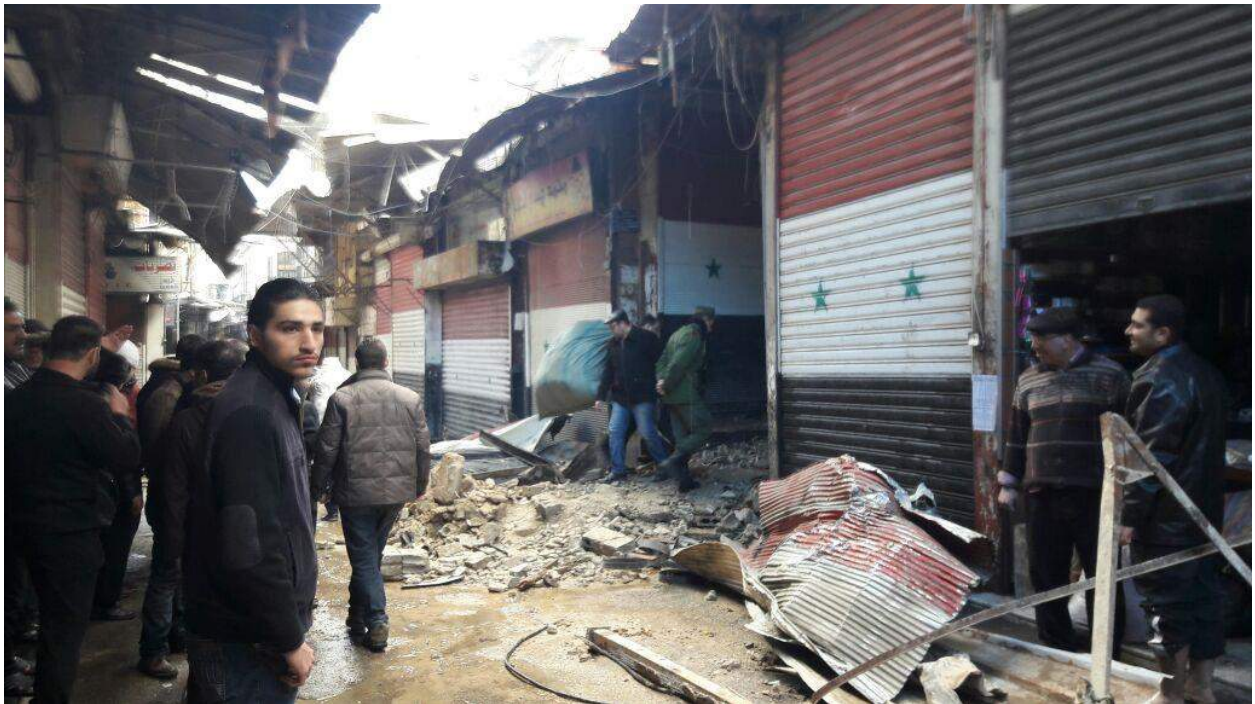
Fire damage in al-Hamidiyah Souq (DGAM; December 2, 2016)
