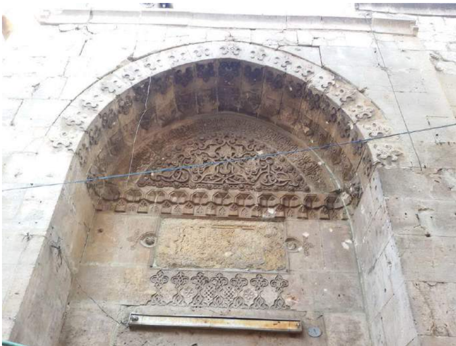
An exterior wall of Bab al-Ahmar Mosque showing bullet damage (Private Facebook Account; December 10, 2016)
