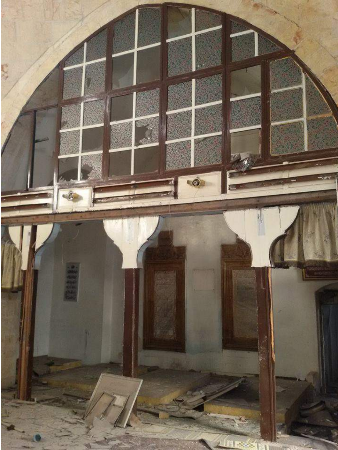
Minor damage to the Musa bin Nasir Madrassa showing missing glass panes and rubble (Private Facebook Account; December 10, 2016)
