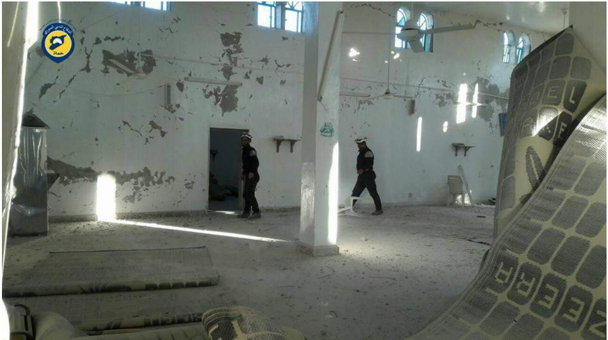
Damage to ceiling of Abu Bakr al-Sidiq Mosque (Hama Civil Defense/Twitter; December 6, 2016)
