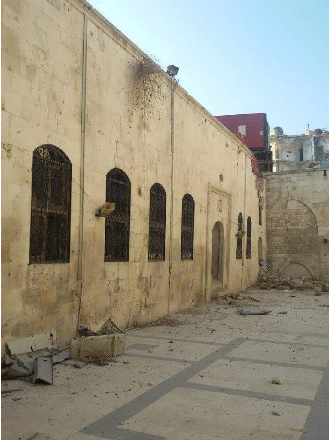
One wall of al-Hadadeen Mosque with less damage to the facade (Private Facebook Account; December 10, 2016)
