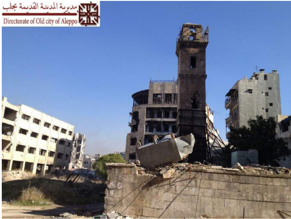
Debris on the wall around Mosque Dabbagha al-'Atiqa and visible damage to the minaret (DGAM; December 9, 2016)
