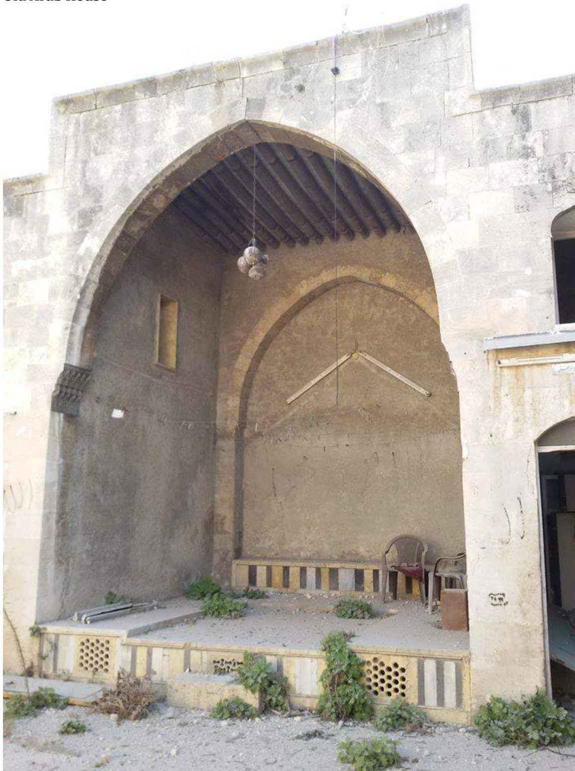
Slight damage to the courtyard of the Old Arab House (Private Facebook Account; December 10, 2016)
