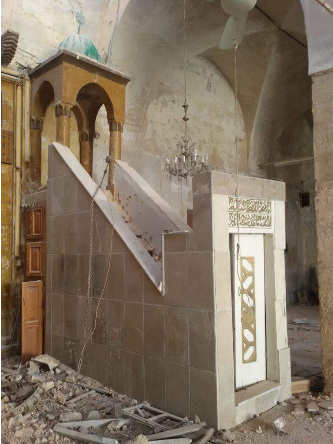
Damage to the minbar at Banqusa Mosque (Private Facebook Account; December 10, 2016)
