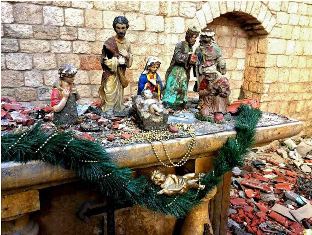
A makeshift nativity scene is set up in the damaged Church of Our Lady (Private Twitter Account; December 8, 2016)
