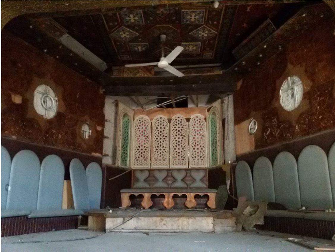
Slight damage to the interior of Hammam Bab al-Ahmar (Private Facebook Account; December 10, 2016)
