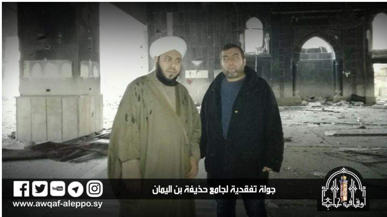
Damage to the interior of Huzeifa ibn al-Yaman Mosque during an inspection of the site (Awqaf Aleppo; December 13, 2016)
