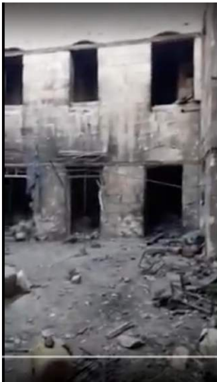
Video still of moderate damage to the Khanqah, showing bullet/shrapnel holes as well as evidence of burning (Khalid Masri; December 12, 2016)
