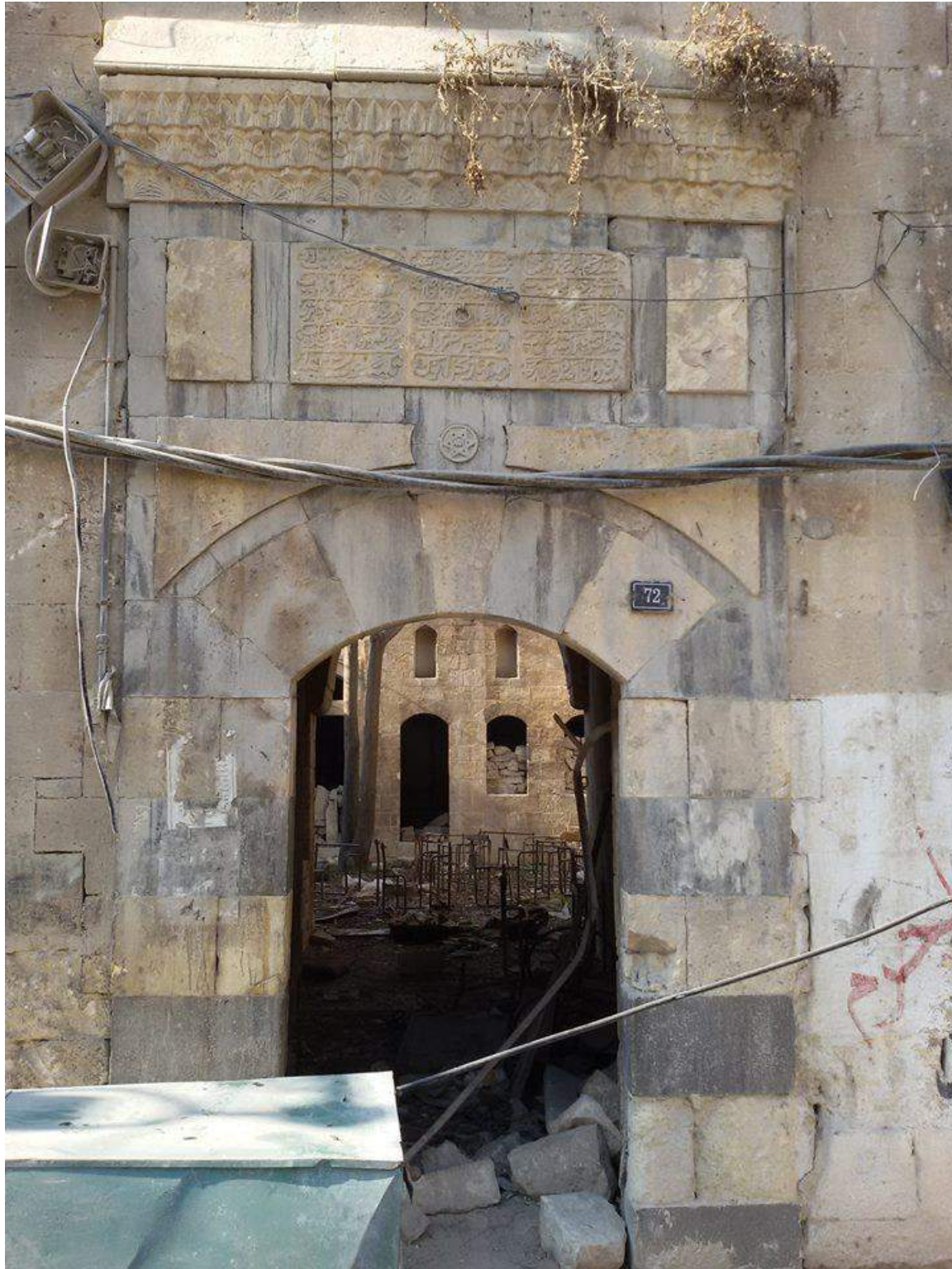
Damage to al-Sarawi Mosque and Madrasa Muqabilat (Private Facebook Account; December 10, 2016)
