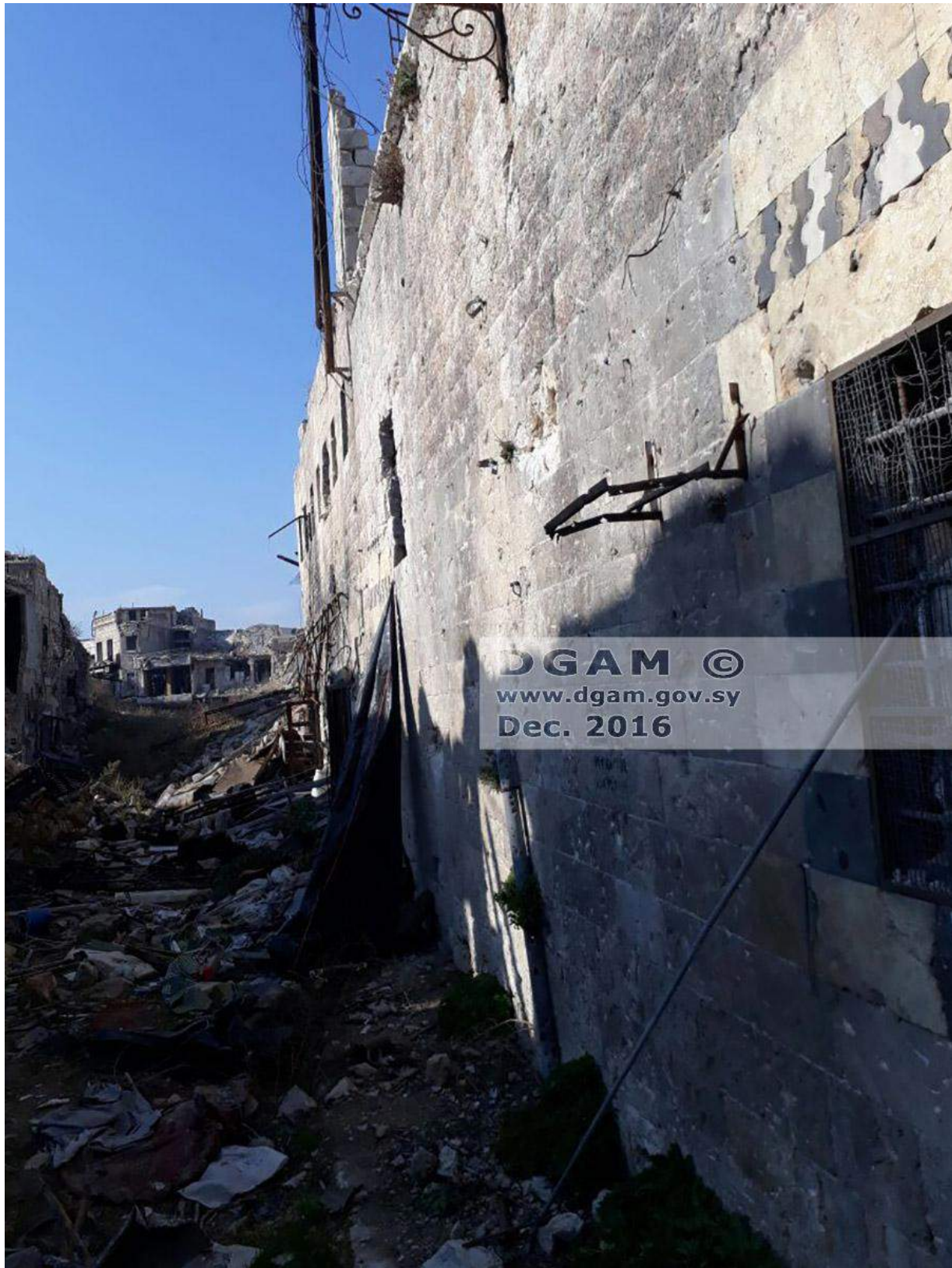
Severe damage to al-Fadileh School (DGAM; December 9, 2016)
