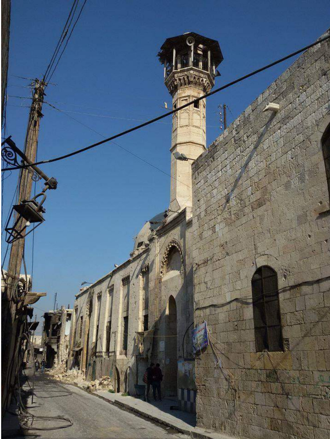
Another view of damage to al-Sarawi Mosque (Private Facebook Account; December 10, 2016)
