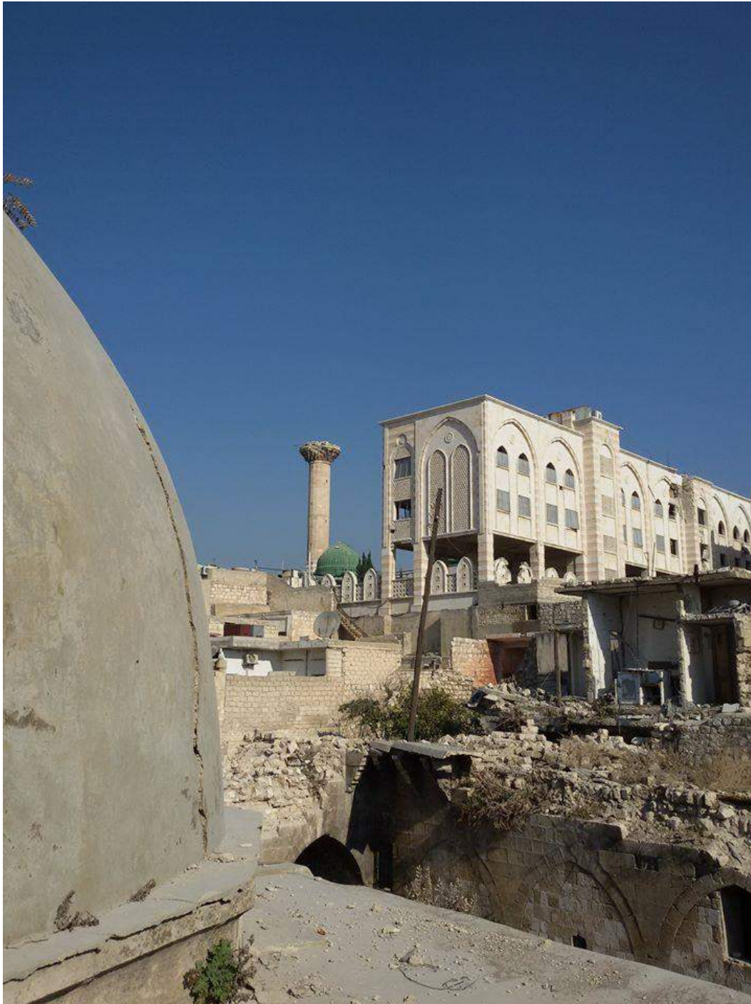
Kiltawiya Madrasa and Mosque in background with green dome and damaged minaret (Private Facebook Account; December 10, 2016)
