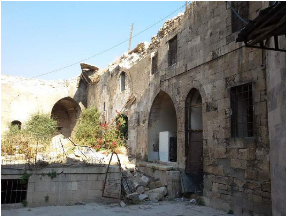
Courtyard of al-Sarawi Mosque showing damage to roof and walls, as well as rubble in courtyard (Private Facebook Account; December 10, 2016)
