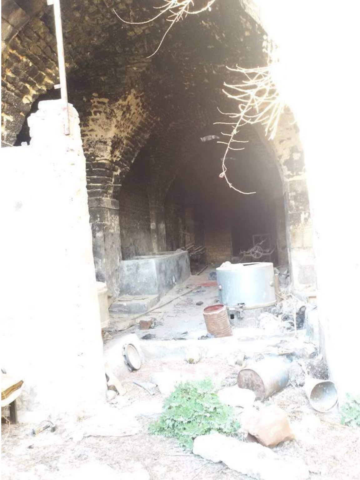
Moderate damage to the interior of Khan Hajj Musa al-Amiri, including evidence of severe burning (Private Facebook Account; December 10, 2016)
