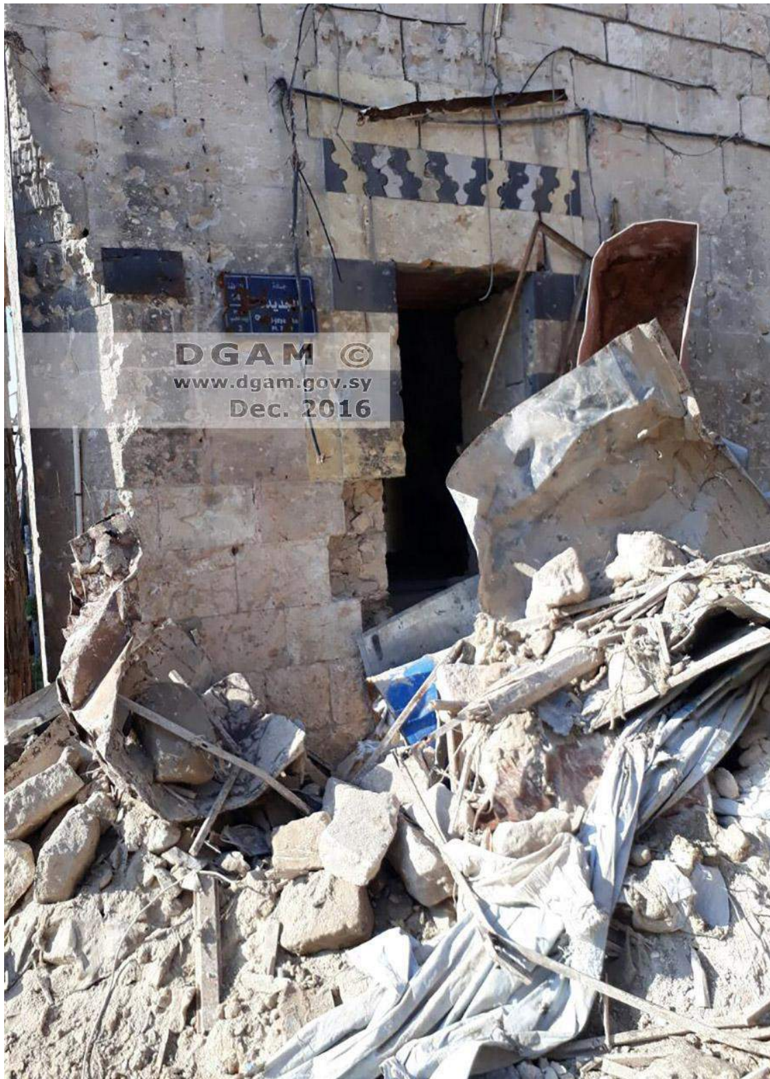
Severe damage to al-Fadileh School (DGAM; December 9, 2016)
