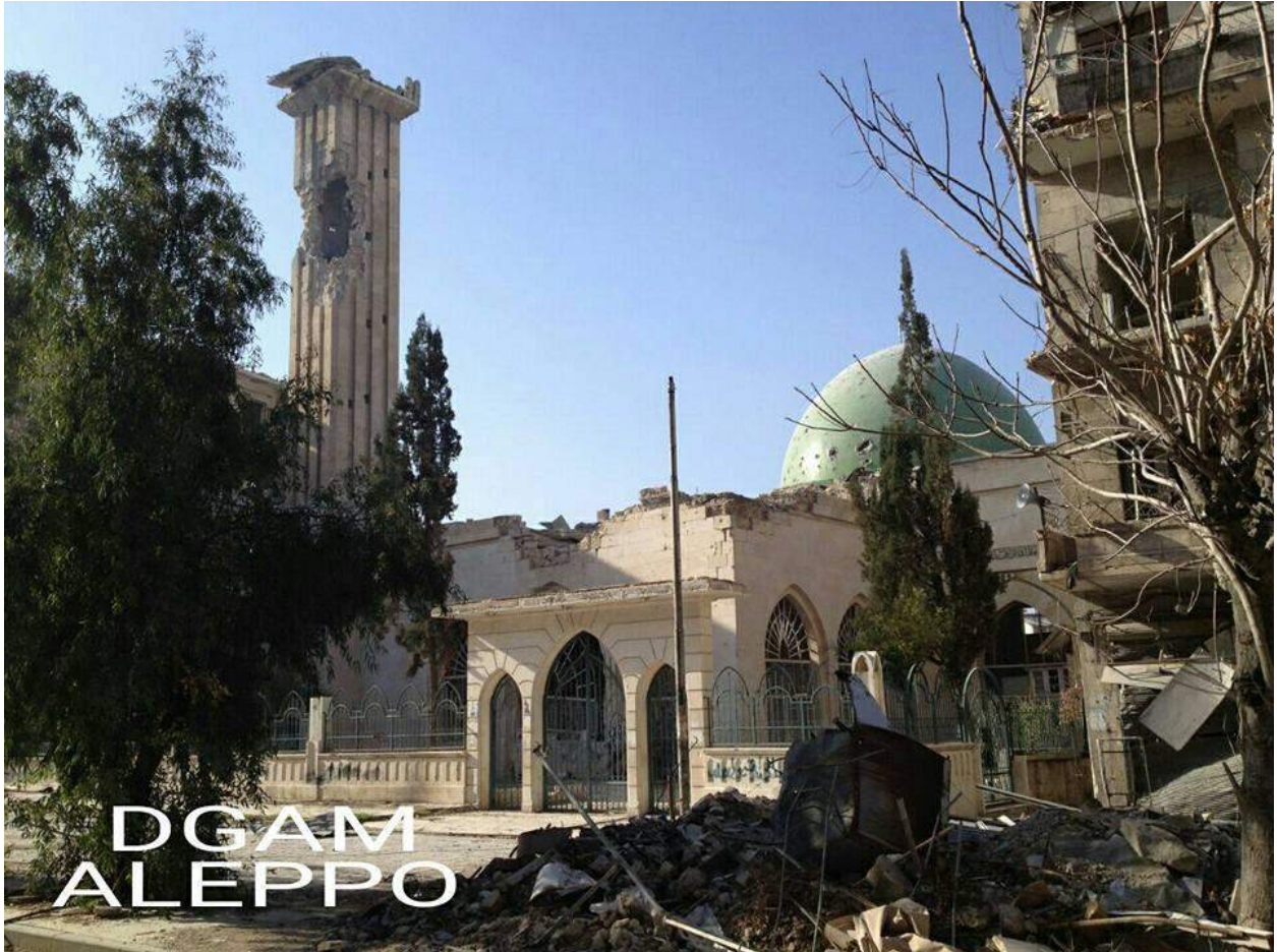
A heavily damaged Usama bin Zaid Mosque in the Old City (Khalid Masri/DGAM; December 9, 2016)
