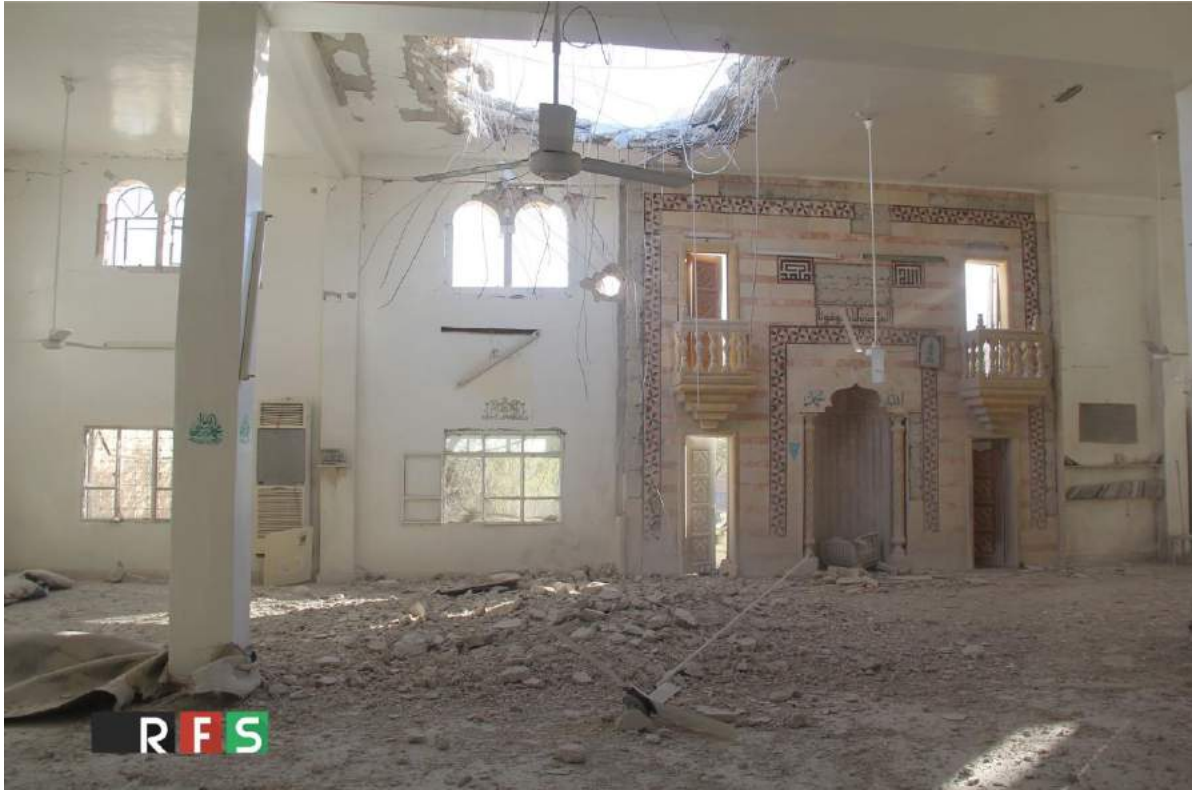
Damage to the ceiling of Abu Bakr al-Sidiq Mosque (RFS Media; December 6, 2016)
