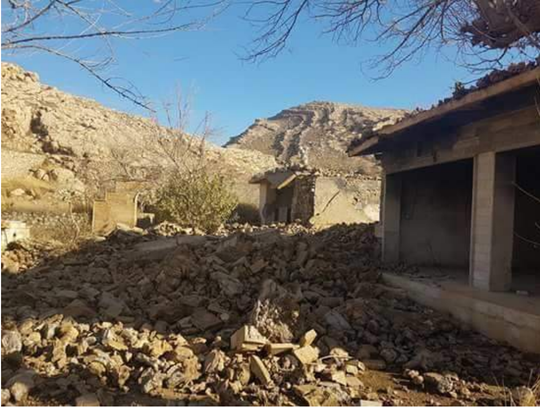
Damage to Sheikh Bakr Shrine (Bahzani and Bashiqa News Events; December 3, 2016)
