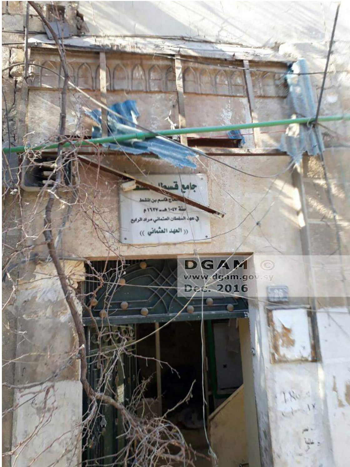
Moderate damage to a building in the Qastal Musht Neighborhood (DGAM; December 9, 2016)
