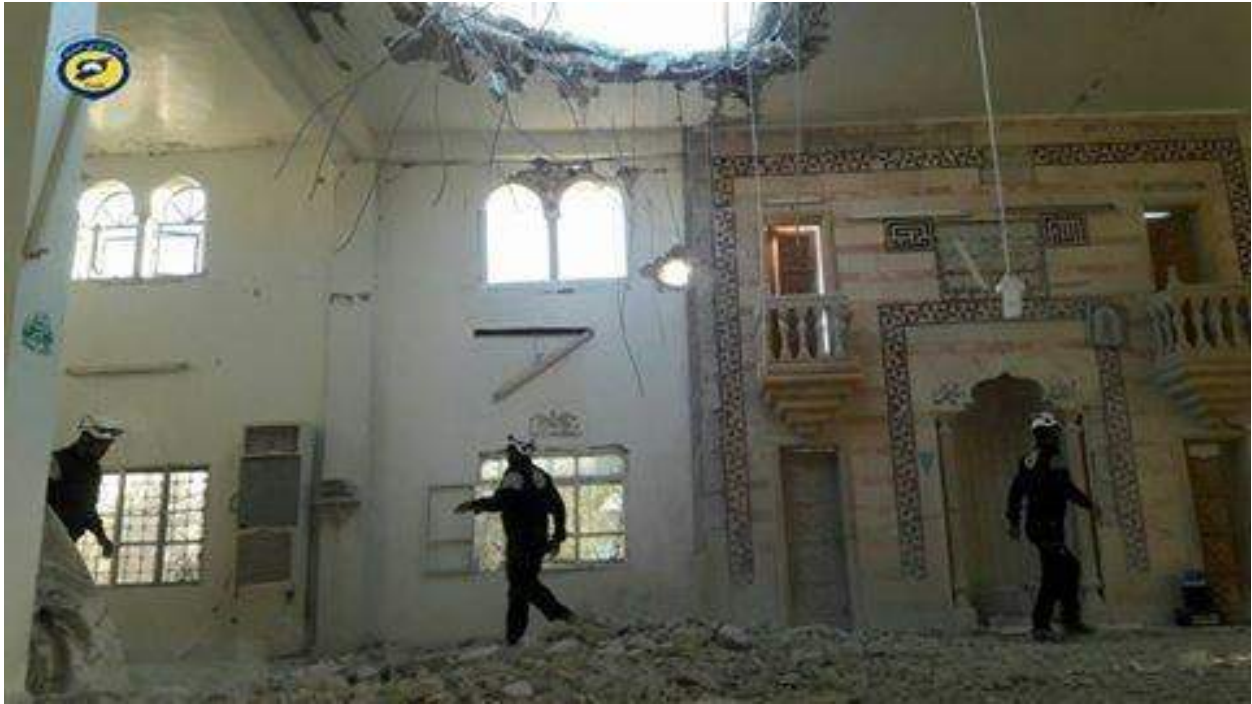
Damage to the ceiling of Abu Bakr al-Sidiq Mosque (Hama Civil Defense/Twitter; December 6, 2016)
