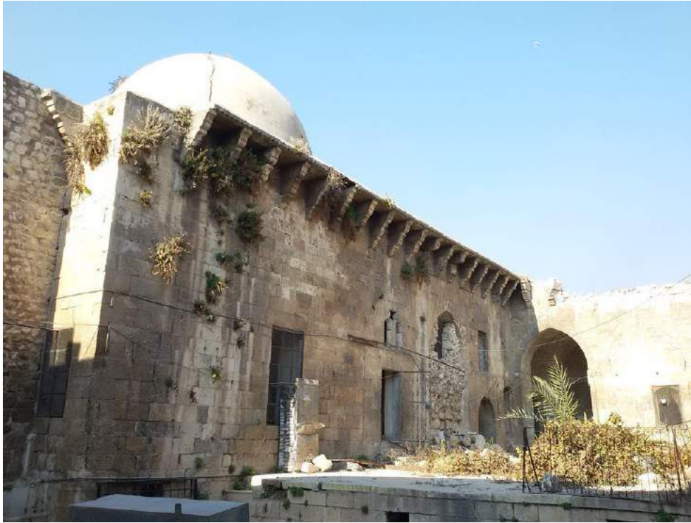
Courtyard of al-Sarawi Mosque showing damage to walls and large crack in dome (Private Facebook Account; December 10, 2016)
