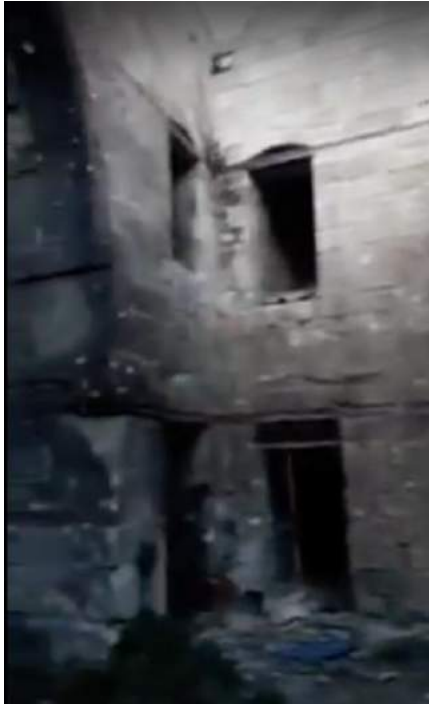
Video still of moderate damage to the Khanqah, showing bullet/shrapnel holes as well as evidence of severe burning (Khalid Masri; December 12, 2016)
