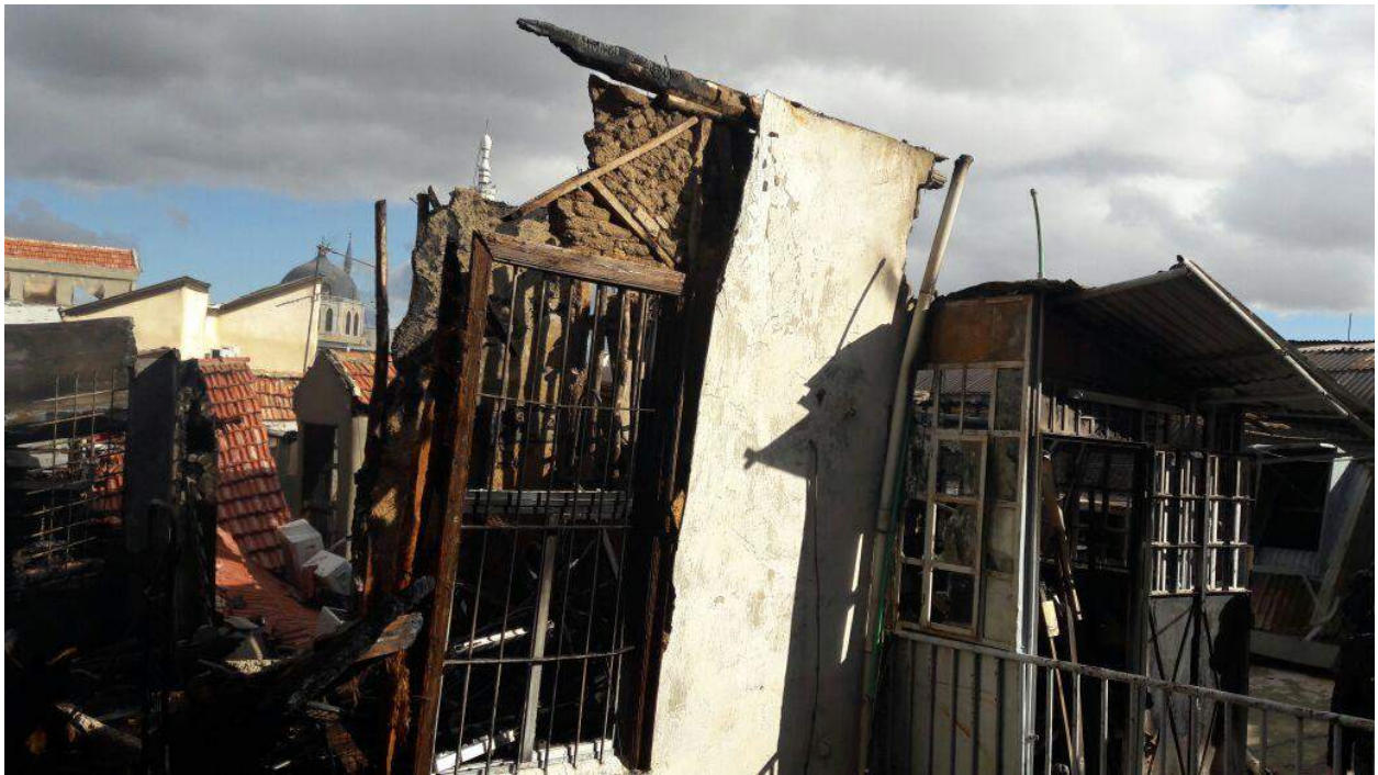
Fire damage in al-Hamidiyah Souq (DGAM; December 2, 2016)
