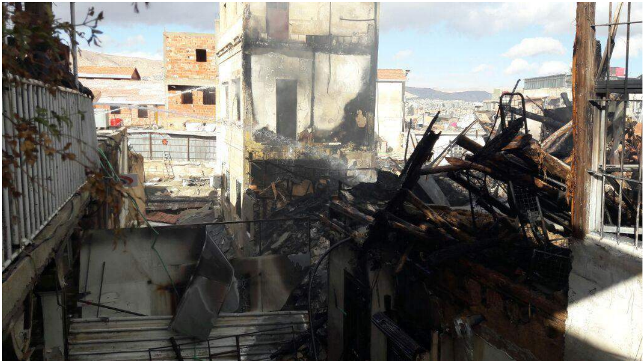
Fire damage in al-Hamidiyah Souq (DGAM; December 2, 2016)
