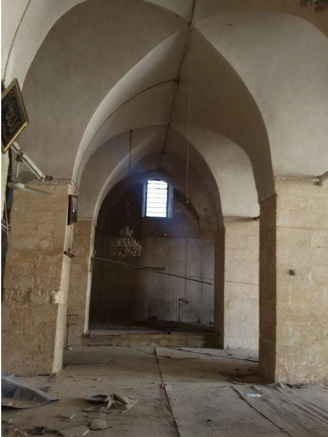
Damage to the interior of Banqusa Mosque (Private Facebook Account; December 10, 2016)
