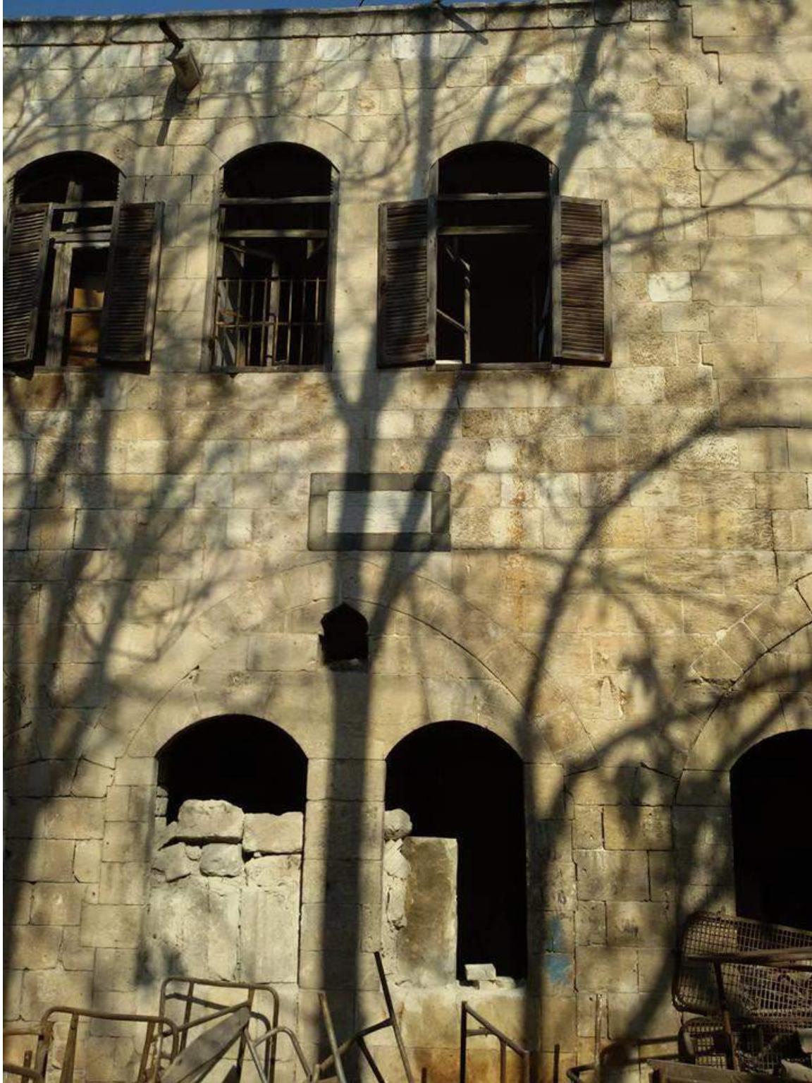
Blocked windows at al-Sarawi Mosque and Madrasa Muqabilat (Private Facebook Account; December 10, 2016)
