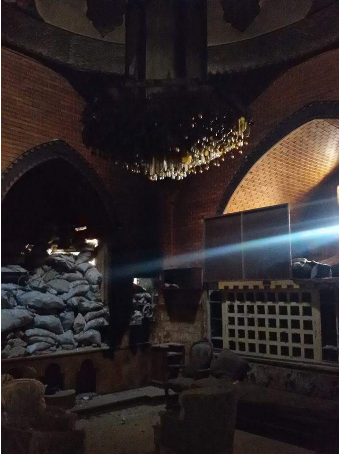
Slight damage to the interior of Hamam Bab al-Ahmar (Private Facebook Account; December 10, 2016)
