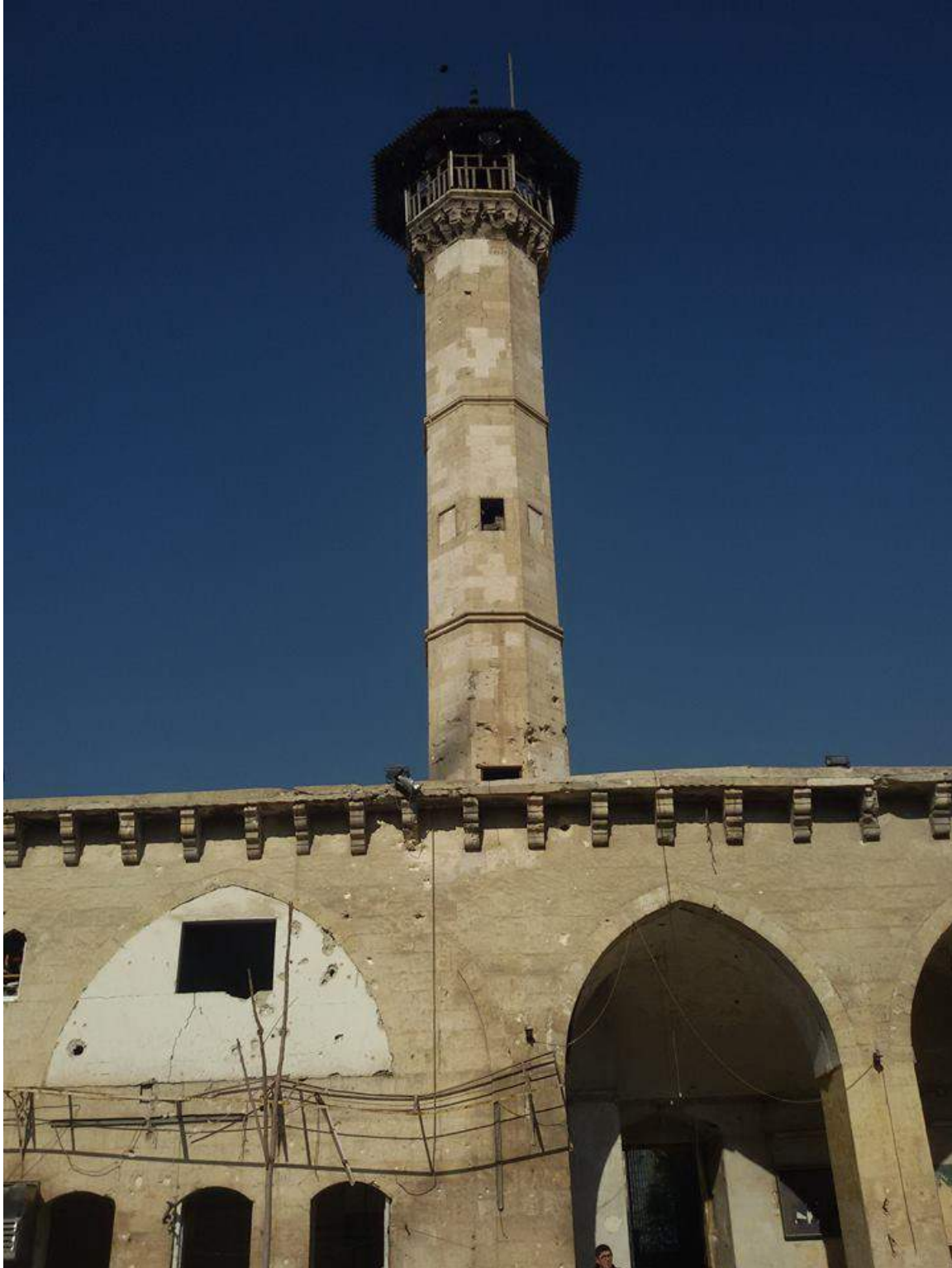
Minaret and walls of Banqusa Mosque showing damage from gunfire/shelling (Private Facebook Account; December 10, 2016)
