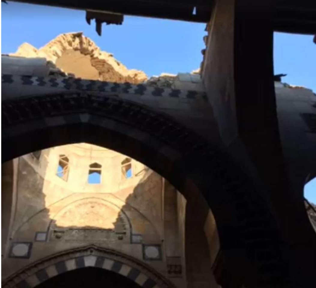
Severe damage to the roof of the Armenian Catholic Church (Armenian.aleppo/Facebook; December 10, 2016)
