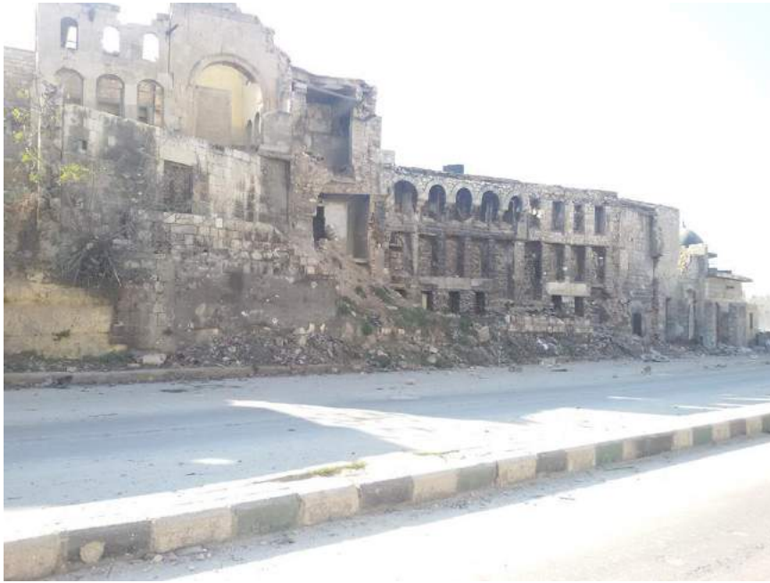
Severe damage to building adjacent to al-Mesla Mosque, with mosque in background (Private Facebook Account; December 10, 2016)
