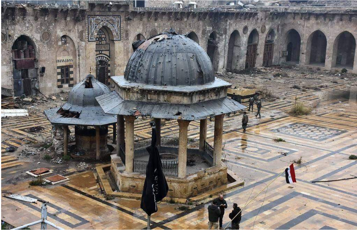
Moderate damage to the structure covering the fountain in the courtyard (Khalid Masri; December 12, 2016)
