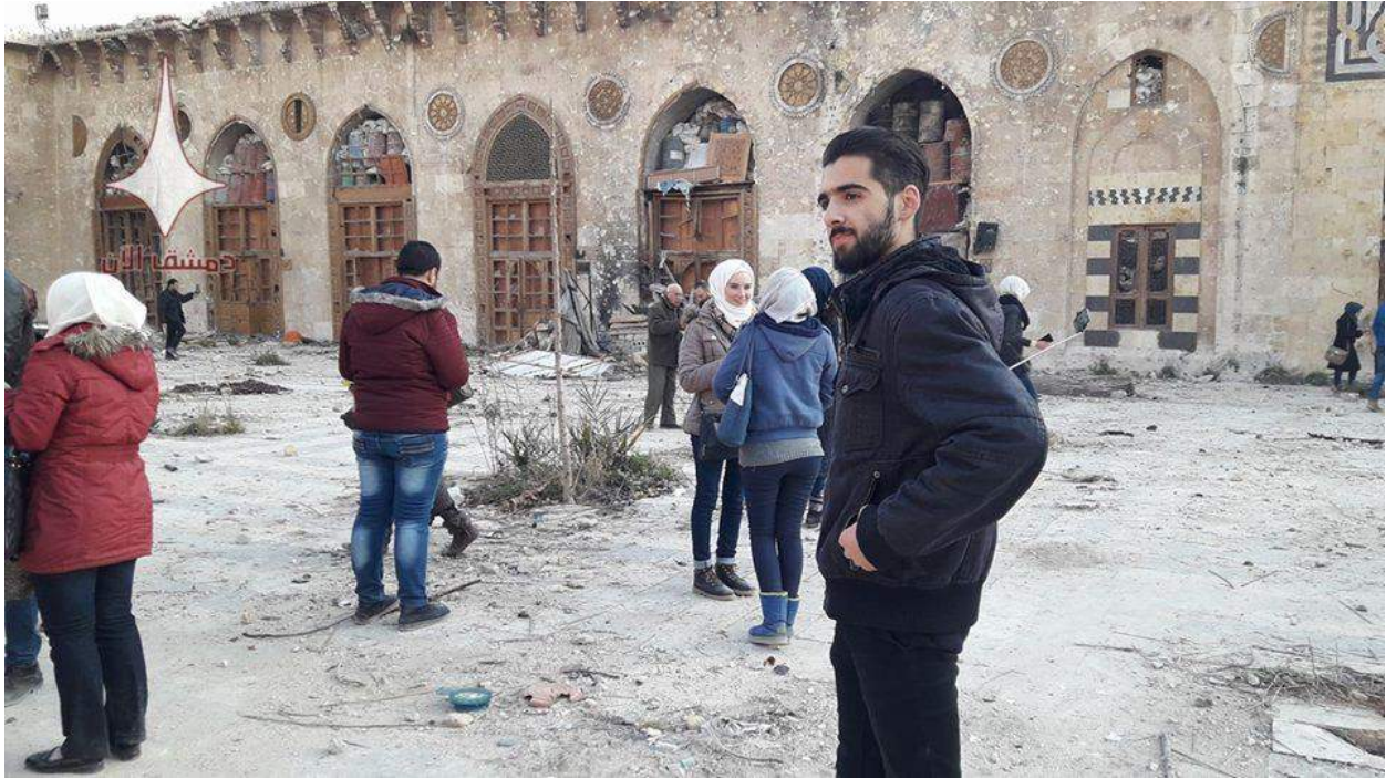
Moderate damage to the Umayyad Mosque courtyard (Aleppo Glory حلب المجد/Facebook; December 10, 2016)
