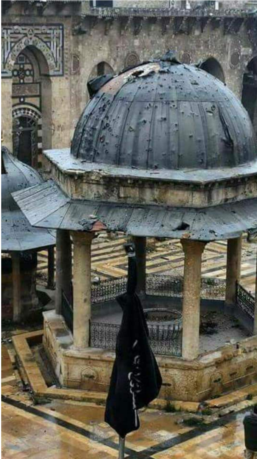
Moderate damage to the structure covering the fountain in the courtyard (Aleppo Glory حلب المجد/Facebook; December 10, 2016)
