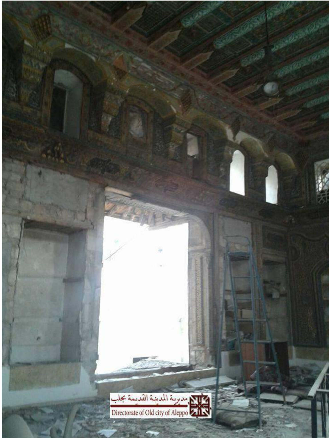
Damage to the interior of Dar Qatar Agassi (Rami M Alafandi; December 12, 2016)
