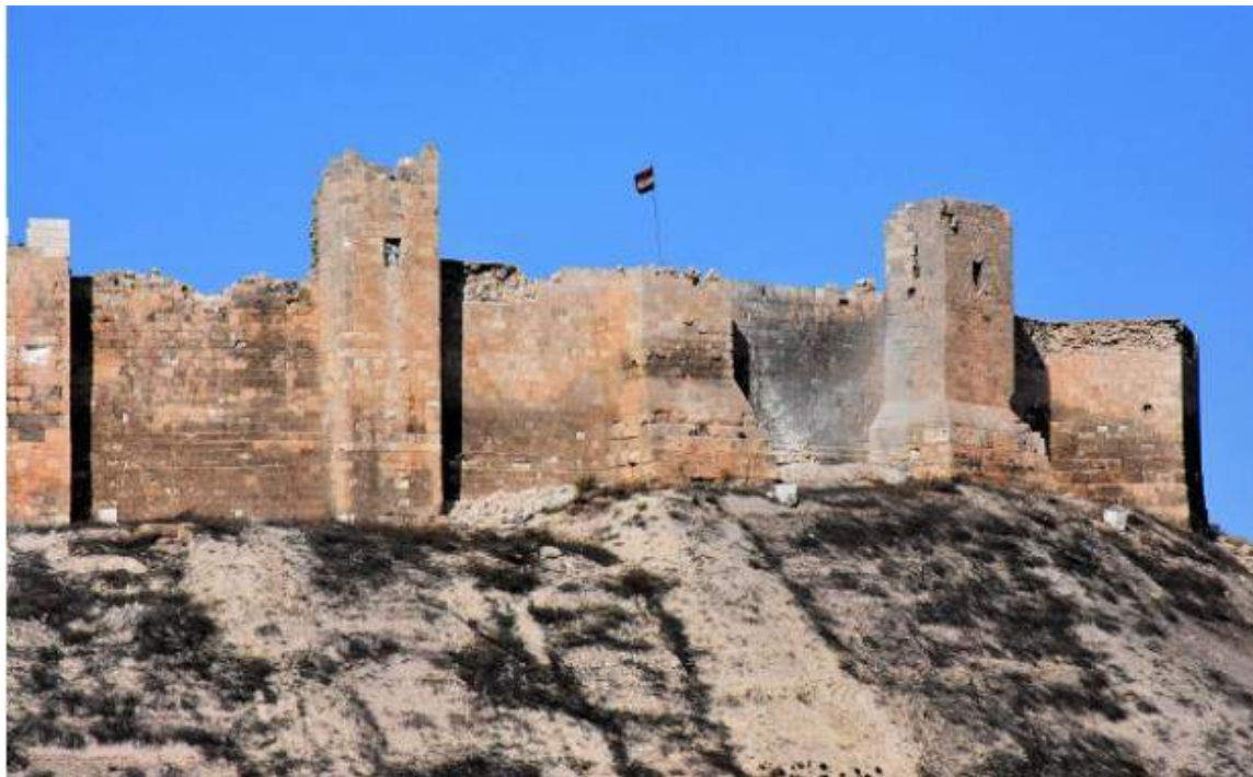
Damage to the Aleppo Citadel (George Ourfalian/AFP; December 8, 2016)
