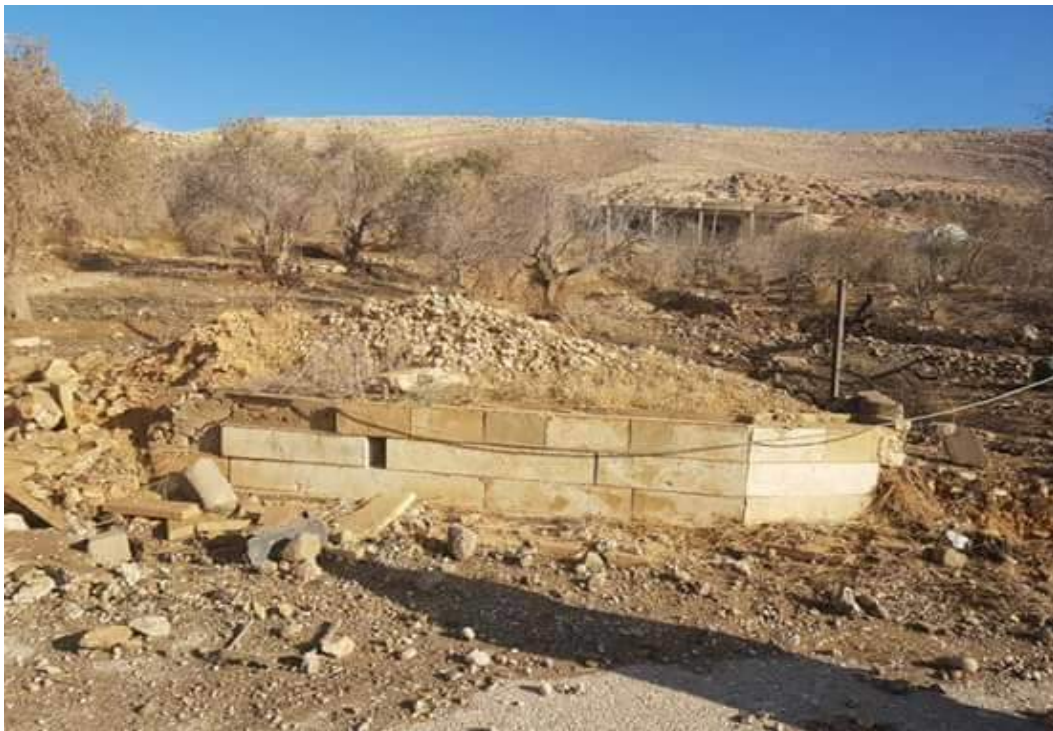
Damage to Sheikh Bakr Shrine (Bahzani and Bashiqa News Events; December 3, 2016)
