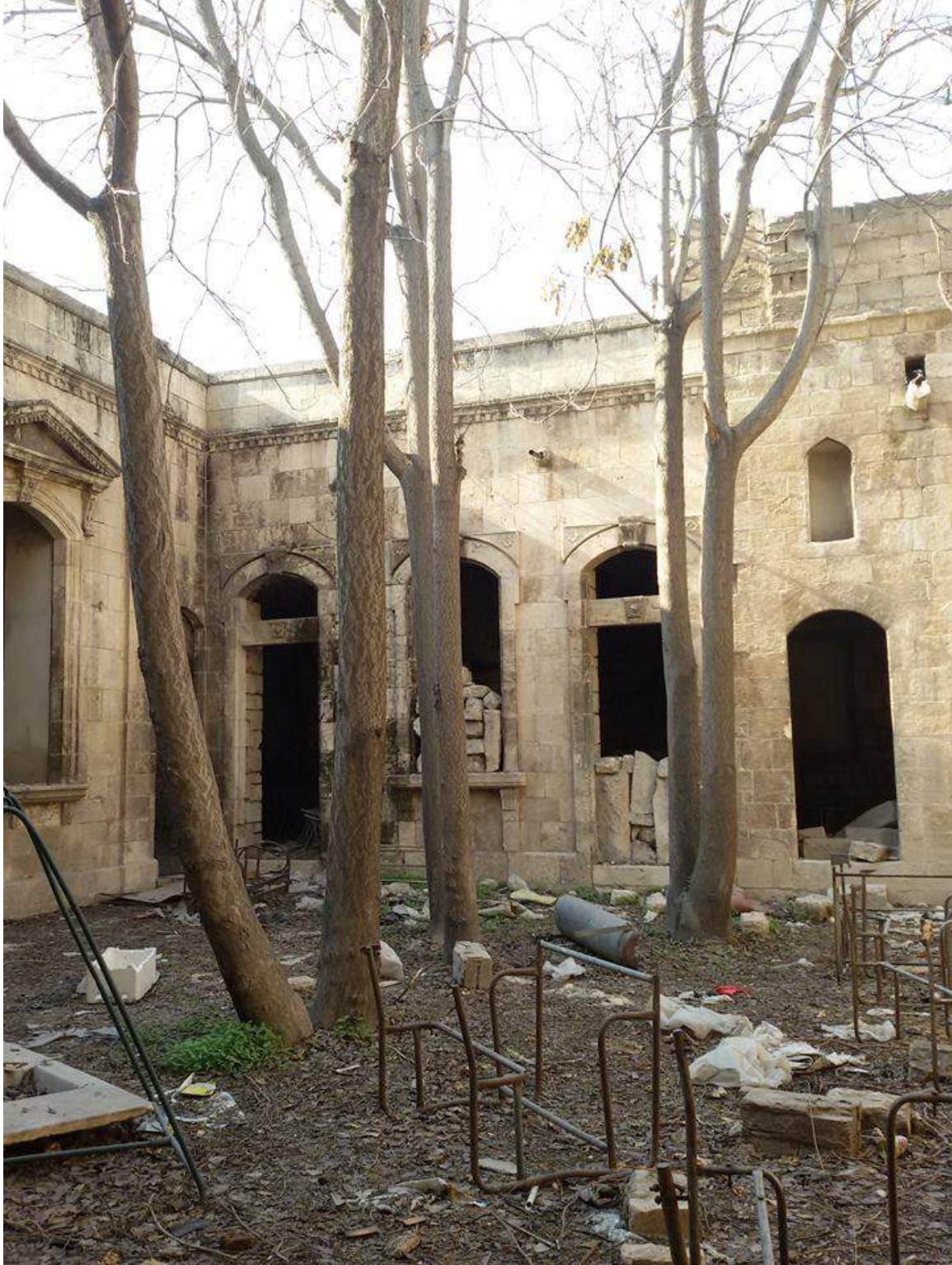
Rubble and debris inside al-Sarawi Mosque and Madrasa Muqabilat (Private Facebook Account; December 10, 2016)
