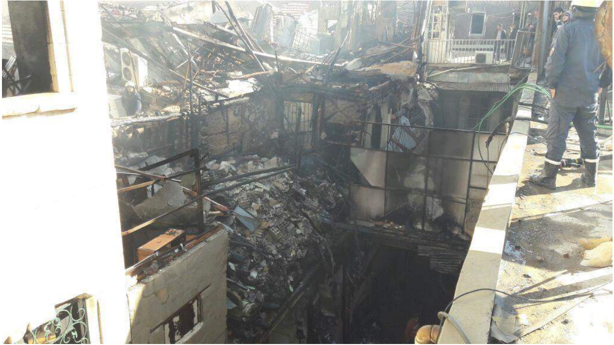
Fire damage in al-Hamidiyah Souq (DGAM; December 2, 2016)
