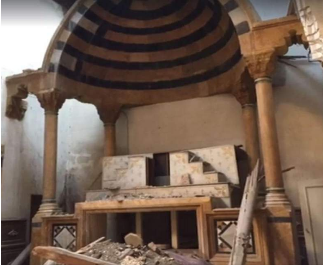
Damage to the altar within the Armenian Catholic Church (Armenian.aleppo/Facebook; December 10, 2016)
