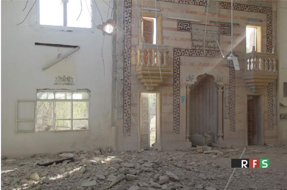
Damage to the interior of Abu Bakr al-Sidiq Mosque (RFS Media; December 6, 2016)
