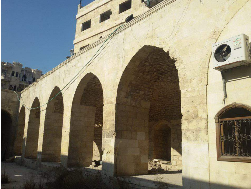
Courtyard of al-Hadadeen Mosque, showing neglect and damage to the structure (Private Facebook Account; December 10, 2016)
