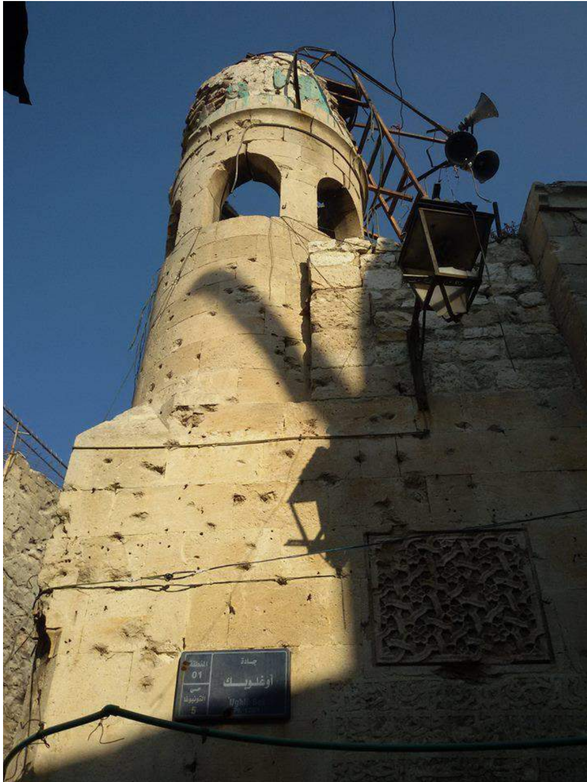
Bab al-Ahmar Mosque with bullet/shrapnel damage and damage to the minaret (Private Facebook Account; December 10, 2016)
