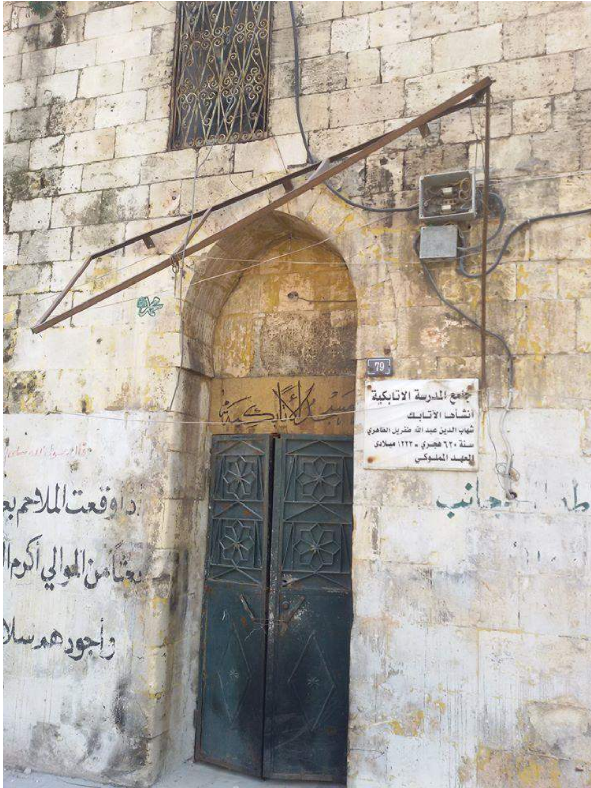
Minor damage to the door of the Atabikiyya Mosque (Private Facebook Account; December 10, 2016)
