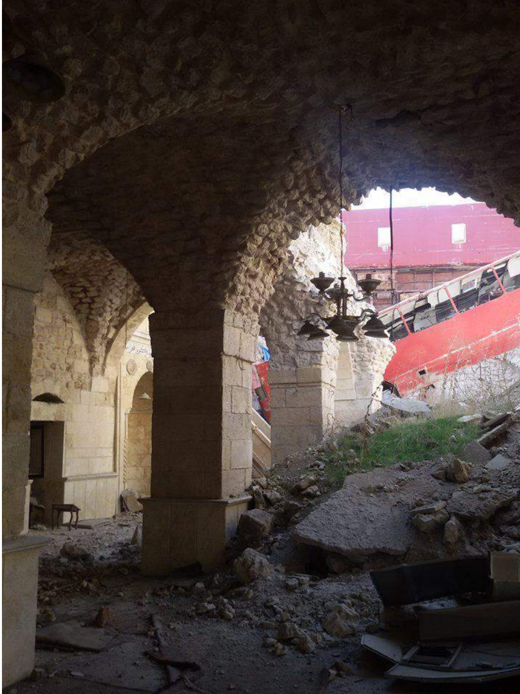
Another view of damage inside al-Hadadeen Mosque, a bus appears wedged alongside the minbar of the mosque (Private Facebook Account; December 10, 2016)
