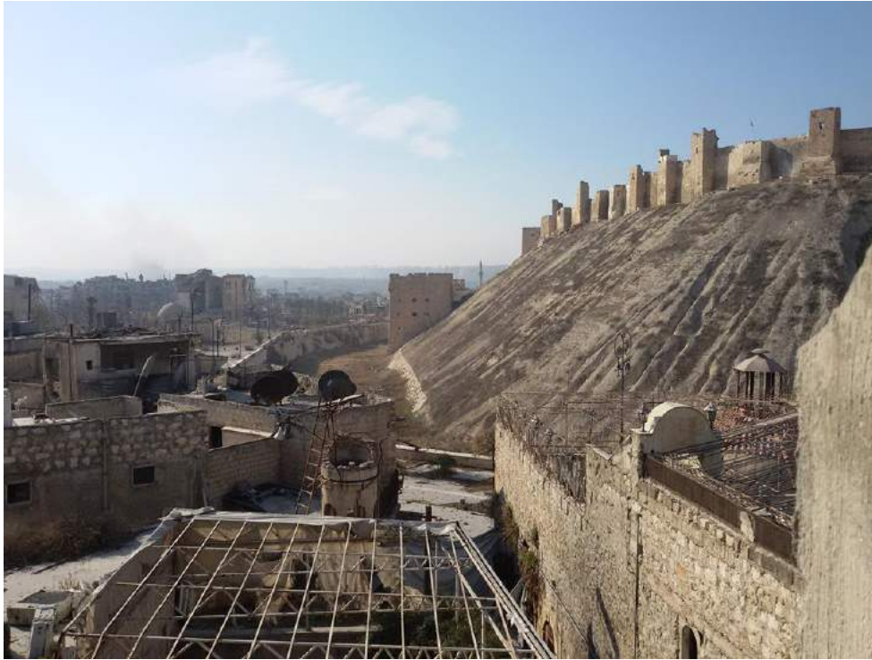
Damage to the roof of Dar al-Fatwa (Private Facebook Account; December 10, 2016)
