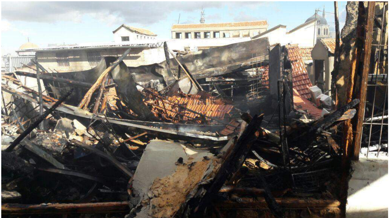
Fire damage in al-Hamidiyah Souq (DGAM; December 2, 2016)
