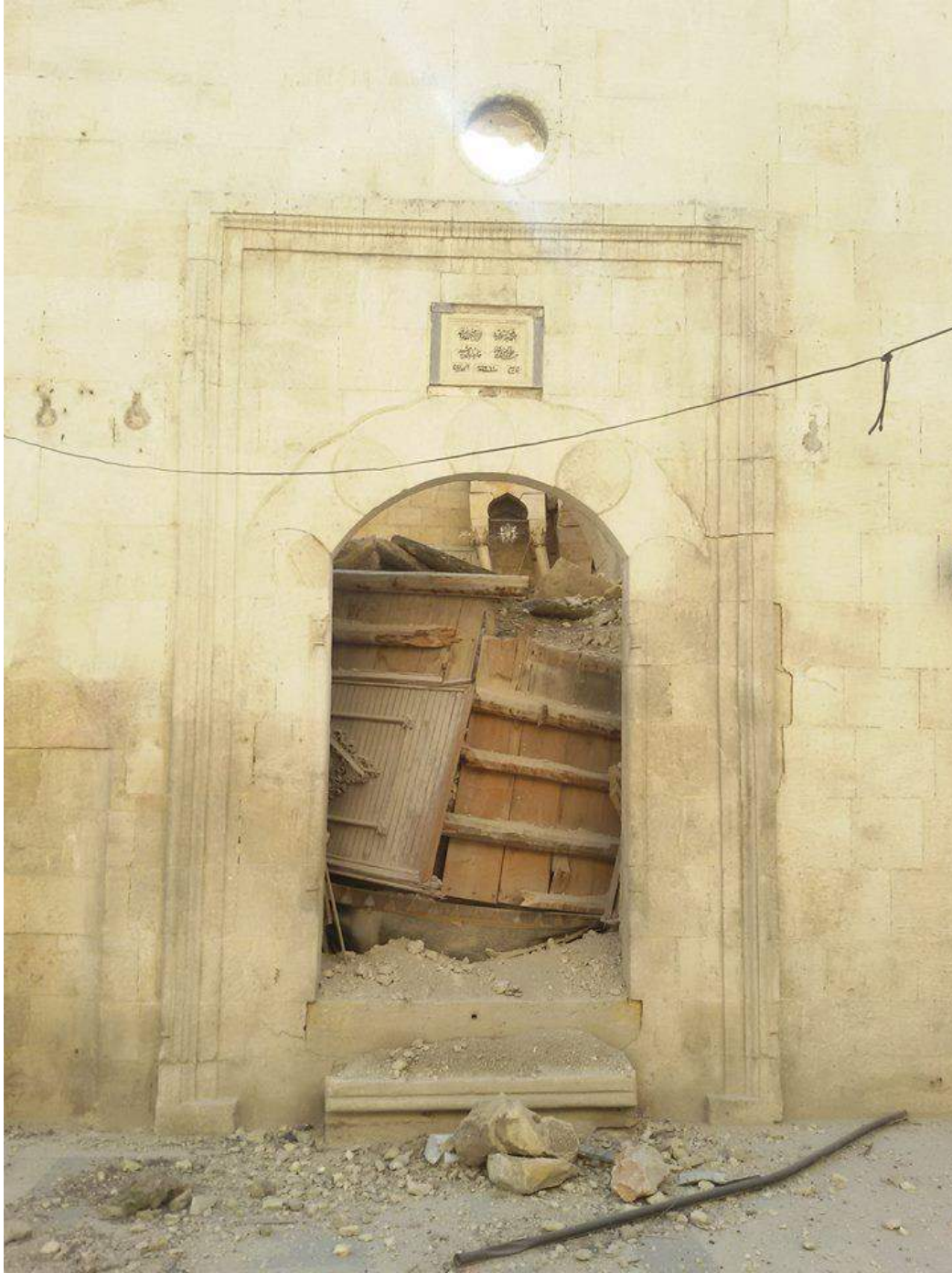
The collapse of what is possibly a ceiling or door inside al-Hadadeen Mosque (Private Facebook Account; December 10, 2016)
