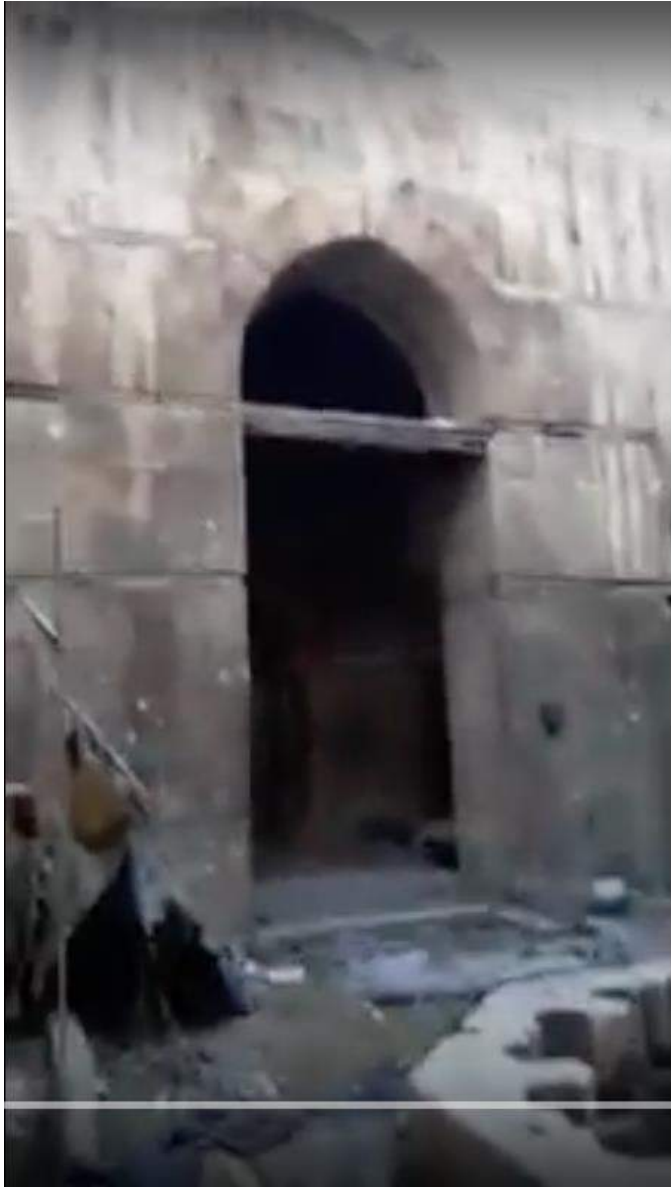
Video still of moderate damage to the Khanqah, showing bullet/shrapnel holes as well as evidence of burning (Khalid Masri; December 12, 2016)
