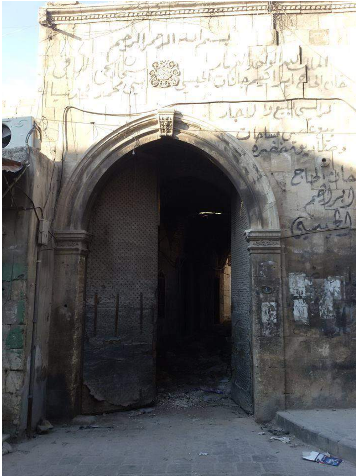
Moderate damage to the entrance of the Khan with evidence of burning and some graffiti (Private Facebook Account; December 10, 2016)
