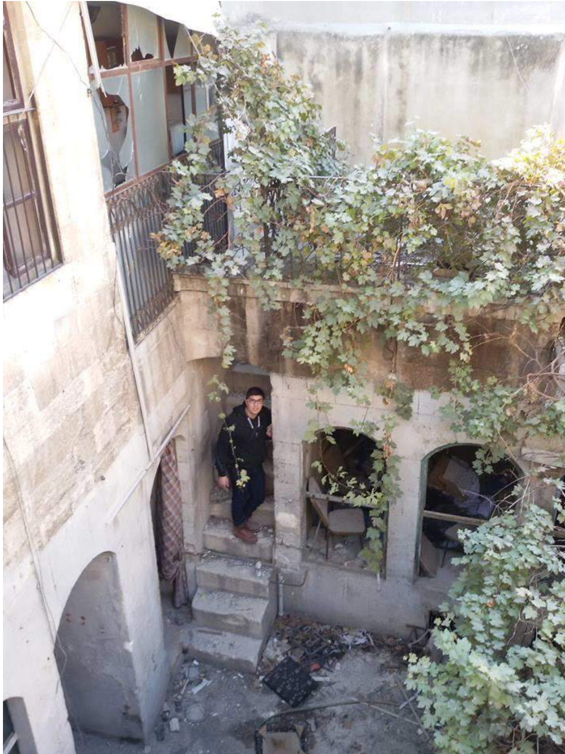
Slight damage to the interior of Hammam Bab al-Ahmar (Private Facebook Account; December 10, 2016)
