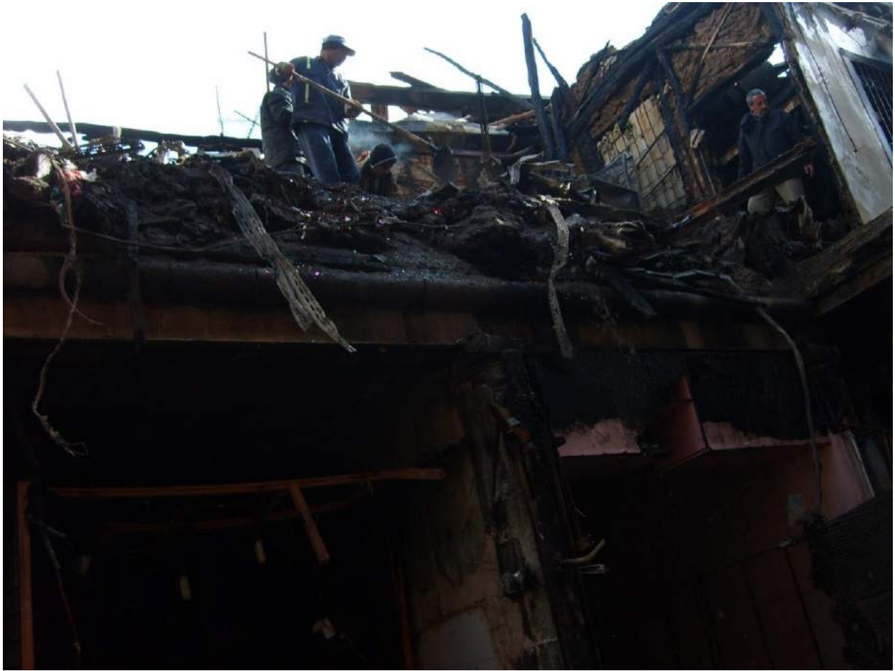
Fire damage in al-Hamidiyah Souq (DGAM; December 3, 2016)
