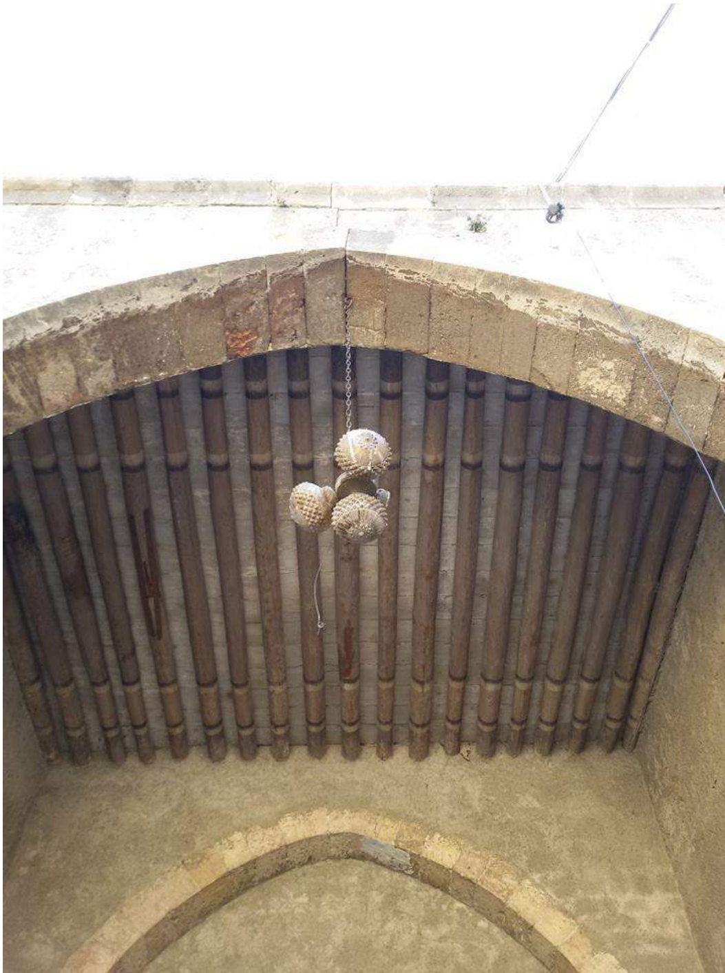
No visible damage to the roof of the old Arab house (Private Facebook Account; December 10, 2016)
