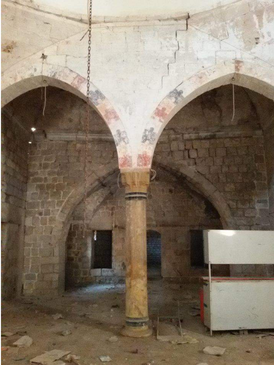
Damage to the inside of al-Sarawi Mosque (Private Facebook Account; December 10, 2016)
