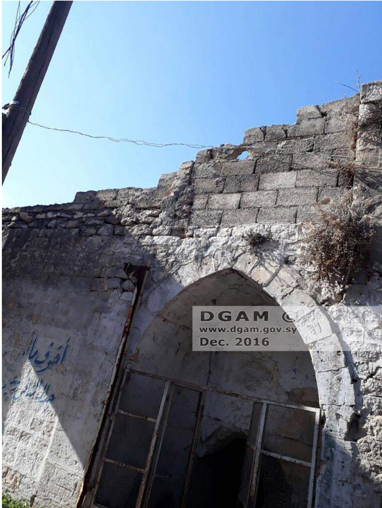
Severe damage to a building in the Qastal Musht Neighborhood (DGAM; December 9, 2016)
