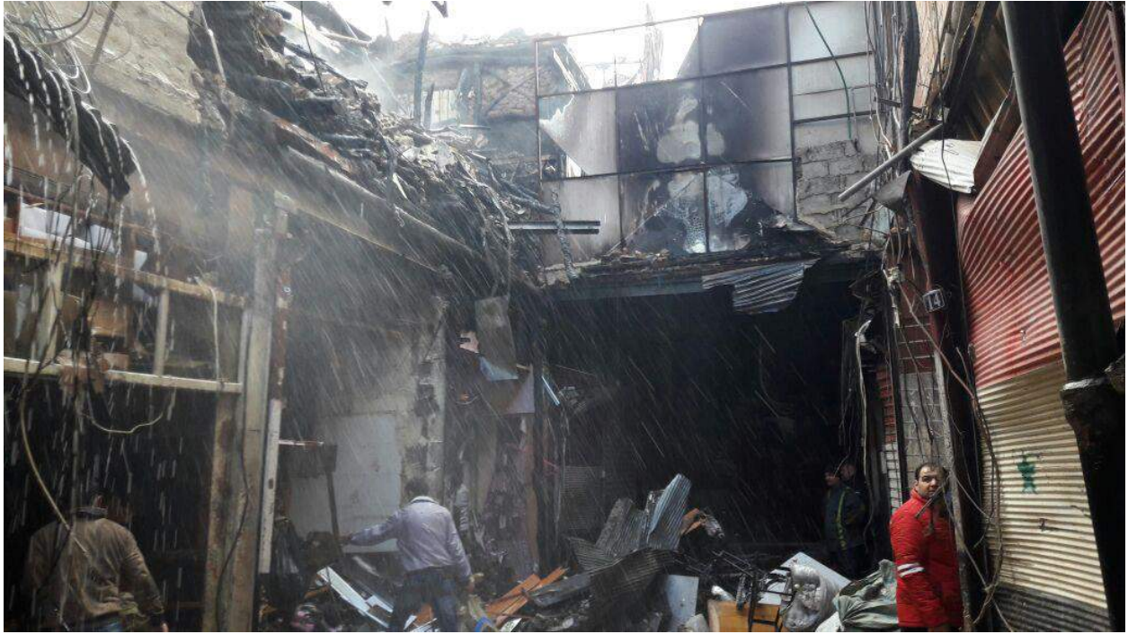
Fire damage in al-Hamidiyah Souq (DGAM; December 2, 2016)
