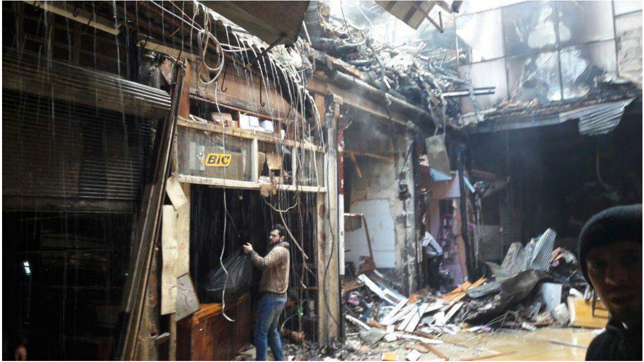
Fire damage in al-Hamidiyah Souq (DGAM; December 2, 2016)
