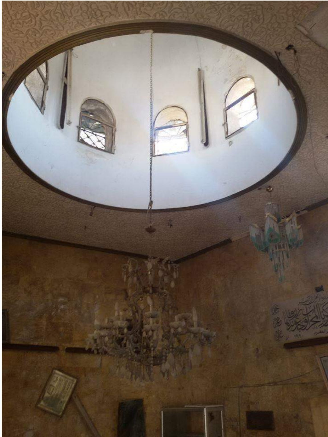
Damage to the interior of al-Mesla Mosque (Private Facebook Account; December 10, 2016)
