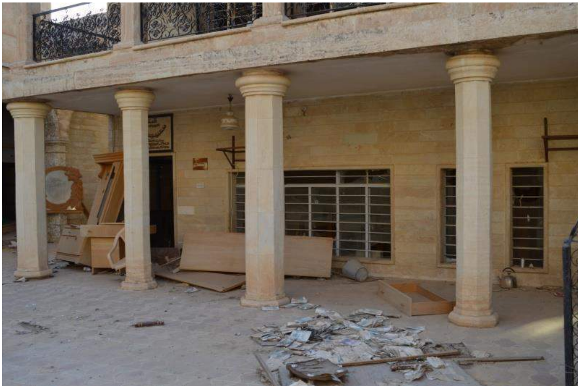
Damage to the complex of Mart Shmone Church (Barely.net; October 22, 2016)
