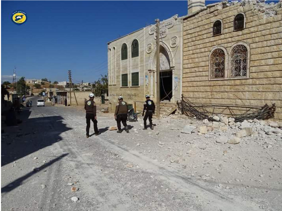
Damage to the exterior of the Grand Tarmala Mosque (The White Helmets; October 20, 2016)
