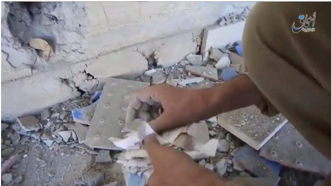
Video still of damage to the interior of al-Shaheeda Mosque (Amaq News Agency; October 16, 2016)
