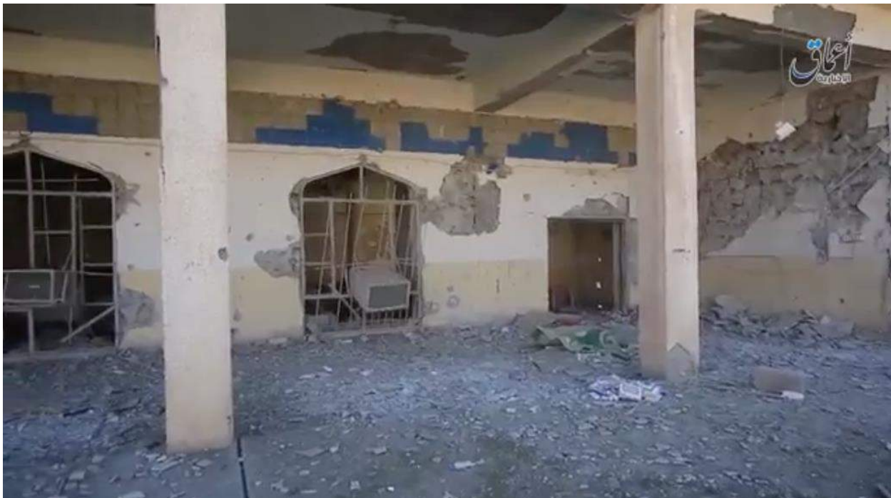
Video still of damage to the exterior of al-Shaheeda Mosque (Amaq News Agency; October 16, 2016)
