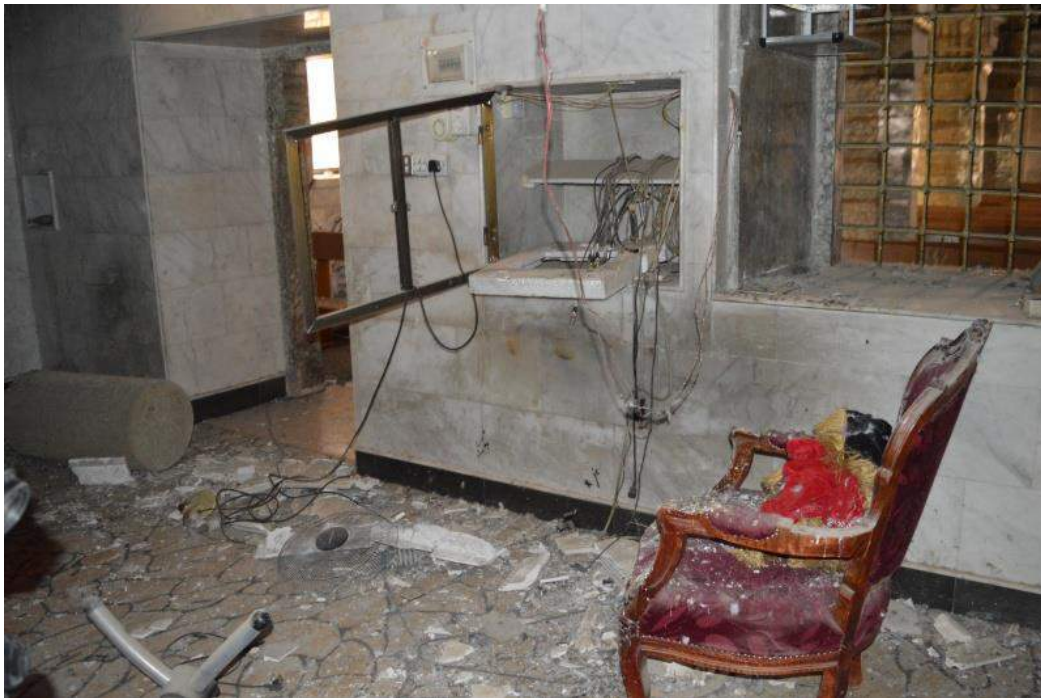
Severe damage to Mart Shmone Church (Baretly.net; October 22, 2016)
