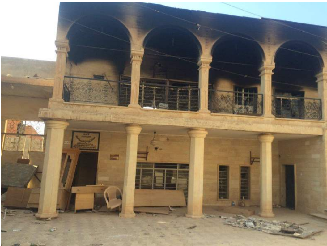
Damage to the complex of Mart Shmone Church (Josie Ensor/Twitter; October 23, 2016)
