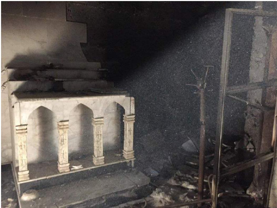
The same damaged altar inside Mart Shmone Church, extensive fire damage is clear (Twitter; October 23, 2016)
