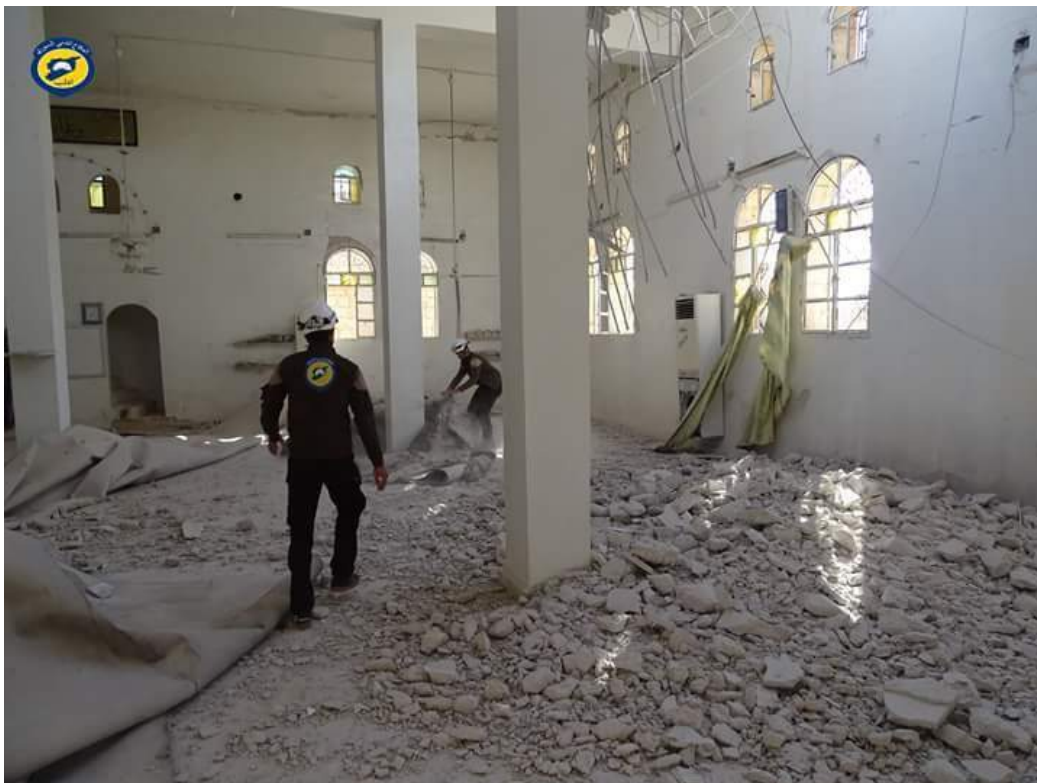
Damage to the interior of the Grand Tarmala Mosque (The White Helmets; October 20, 2016)
