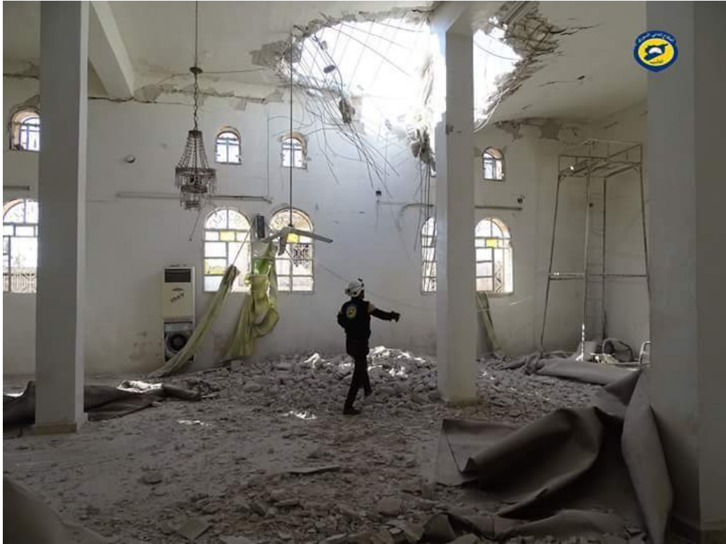
Damage to the interior of the Grand Tarmala Mosque (The White Helmets; October 20, 2016)
