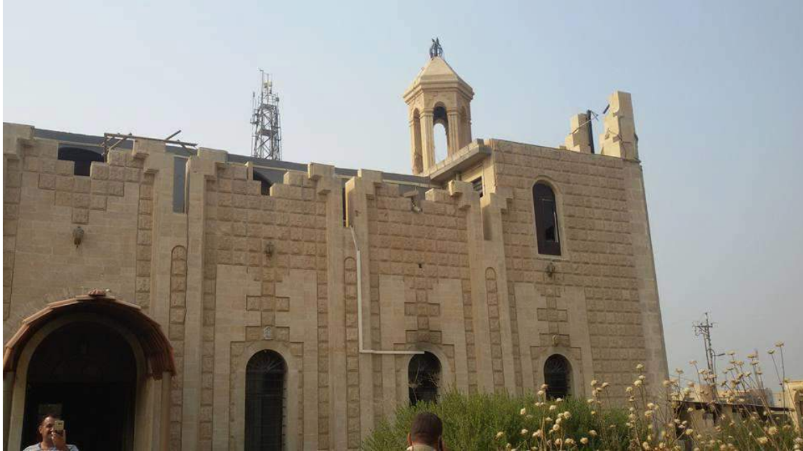
An Exterior wall of Mar Gewargis Church following the recapture of Bartella (Bartella Cafe; October 25, 2016)
