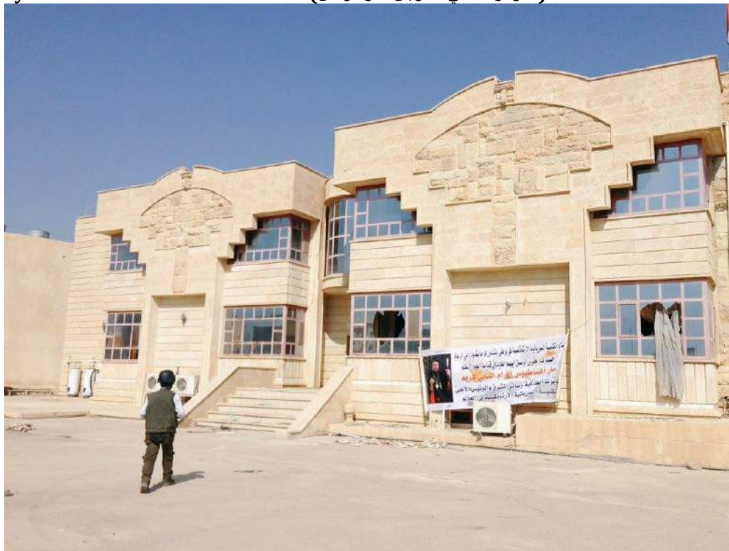
Damage to the Syriac Orthodox Cultural Center (October 24, 2016)
