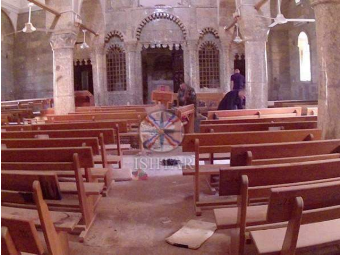
Damage to the interior of Maryam al-Azra Church (Bartella Cafe; October 25, 2016)
