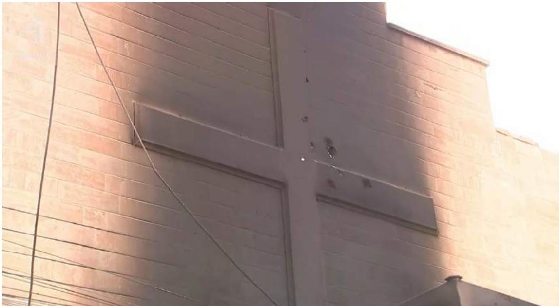
Video still of bullet holes and fire damage outside Maryam al-Azra Church (Channel 4; October 23, 2016)
