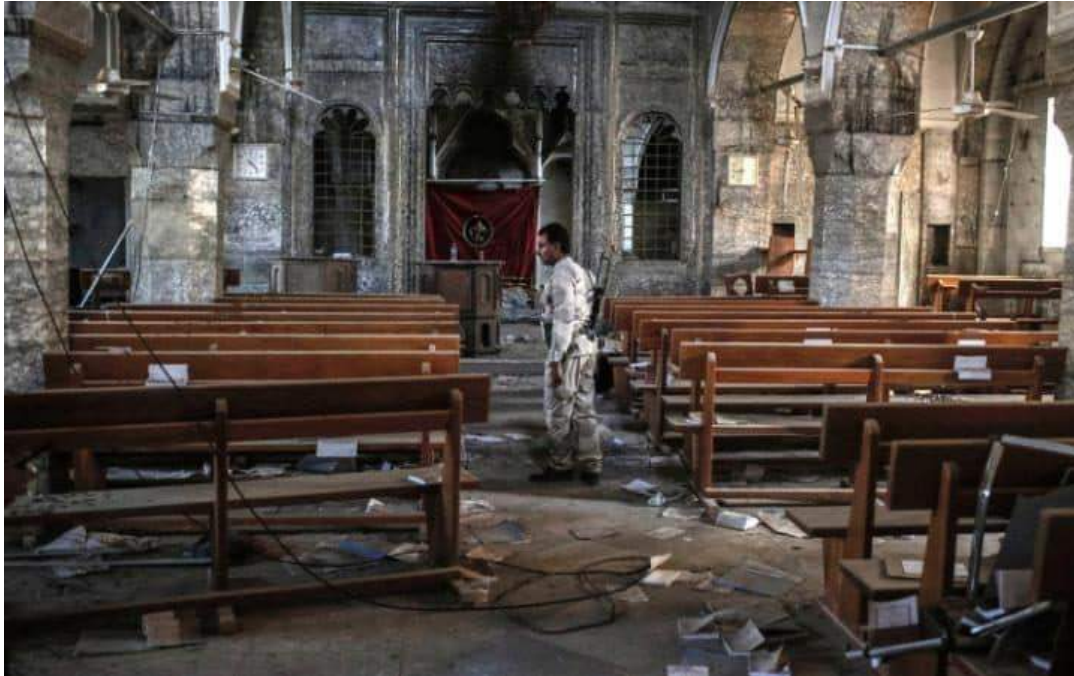
Damage to the interior of Mart Shmone Church (Telegraph; October 21, 2016)
