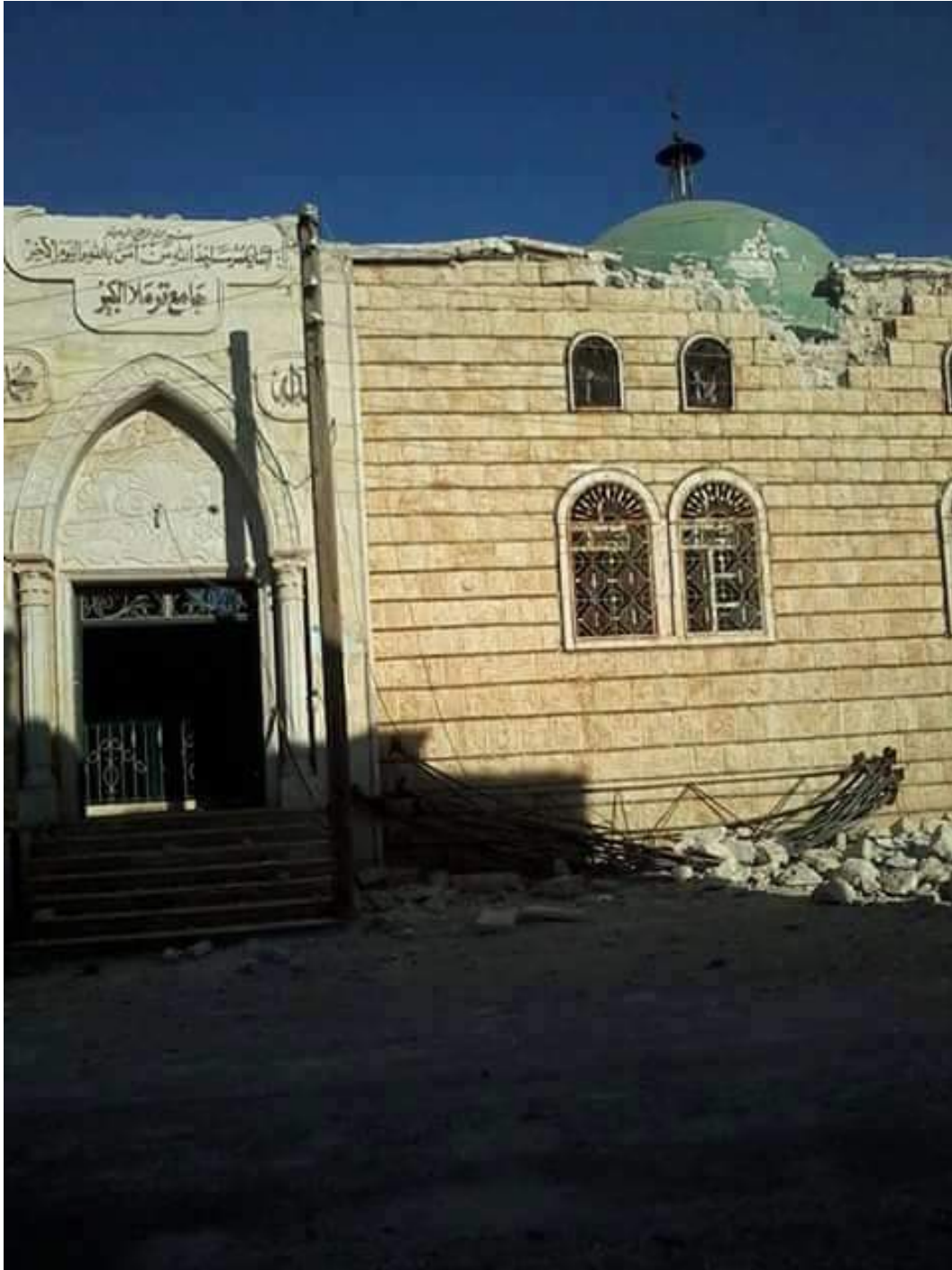
Damage to the Grand Tarmala Mosque (SNHR; October 20, 2016)
