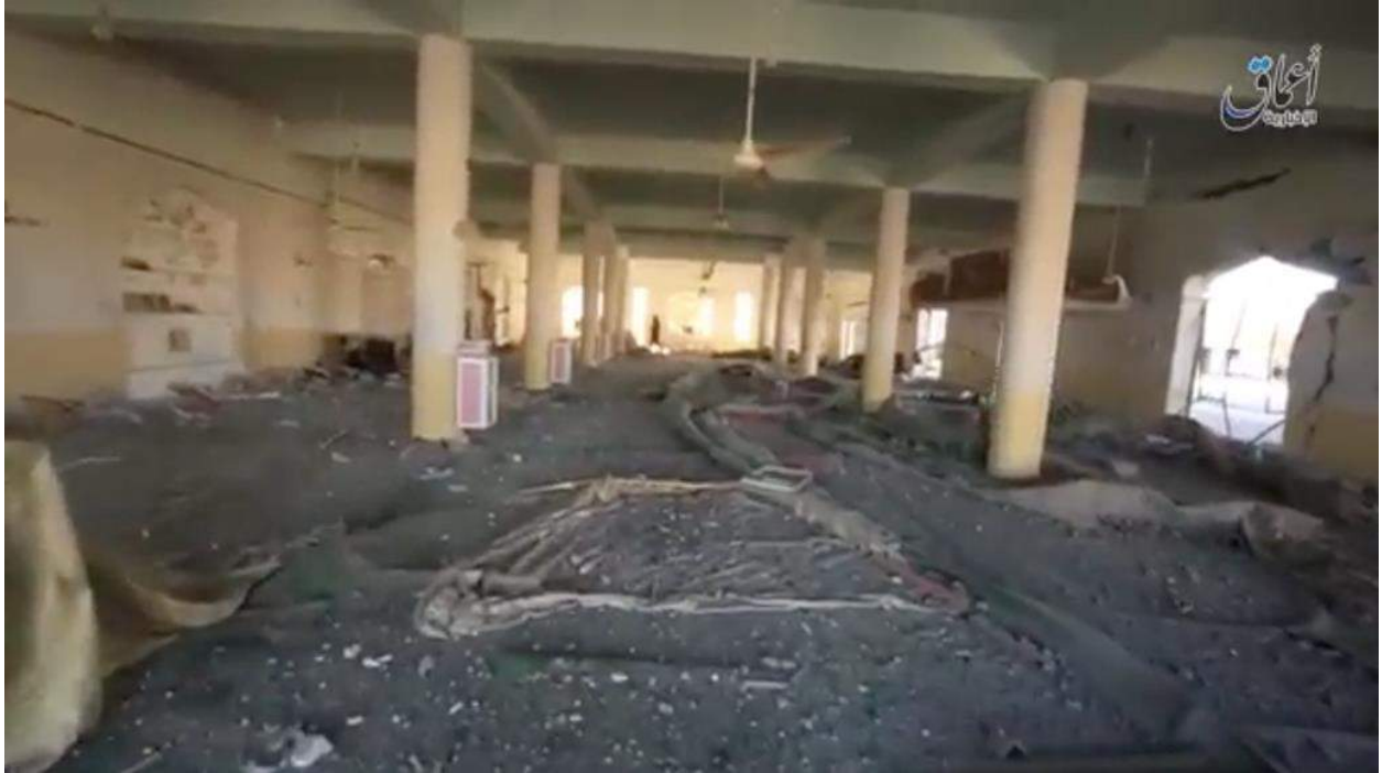
Video still of damage to the interior of al-Shaheeda Mosque (Amaq News Agency; October 16, 2016)
