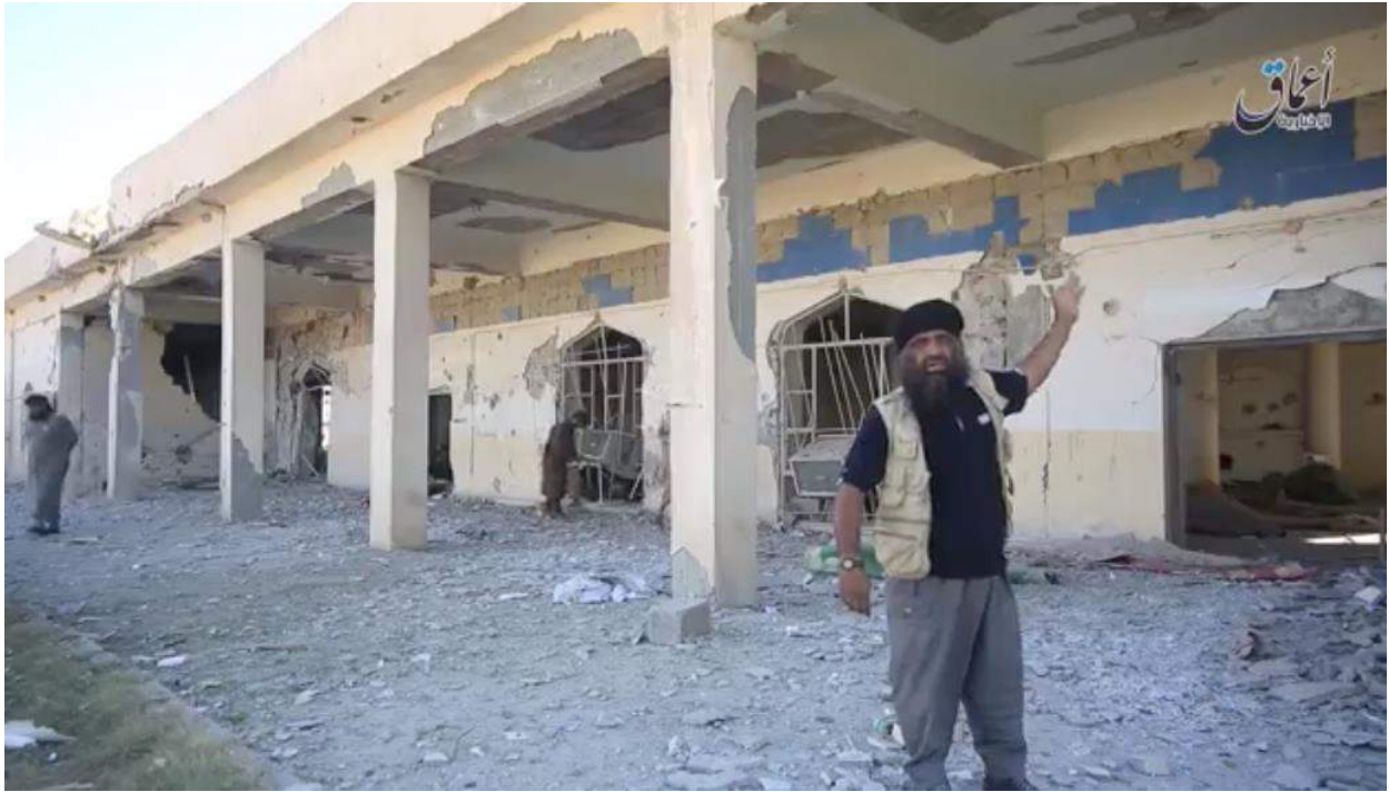
Video still of damage to al-Shaheeda Mosque (Amaq News Agency; October 16, 2016)
