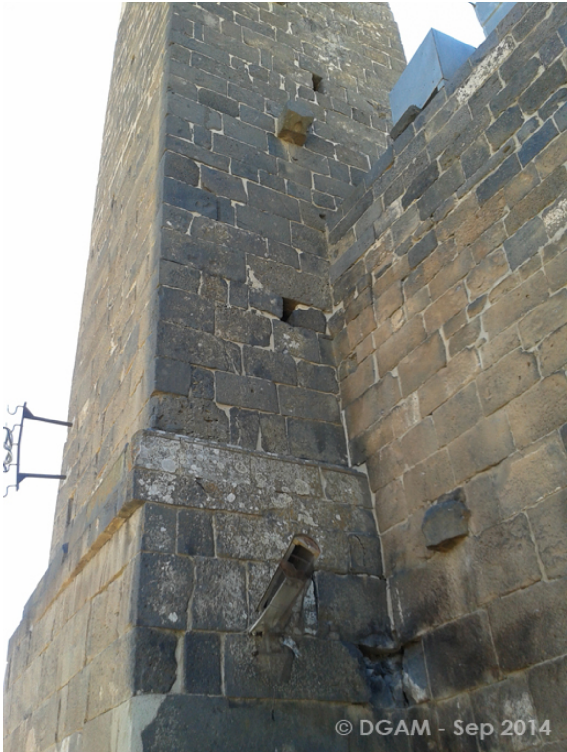
Image of the al-Omari Mosque in the Ancient City of Bosra (DGAM)
