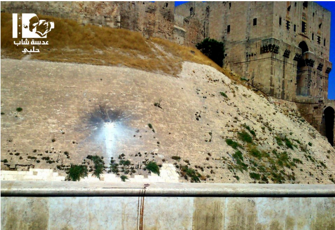
Image showing damage to the Citadel of Aleppo (APSA)
