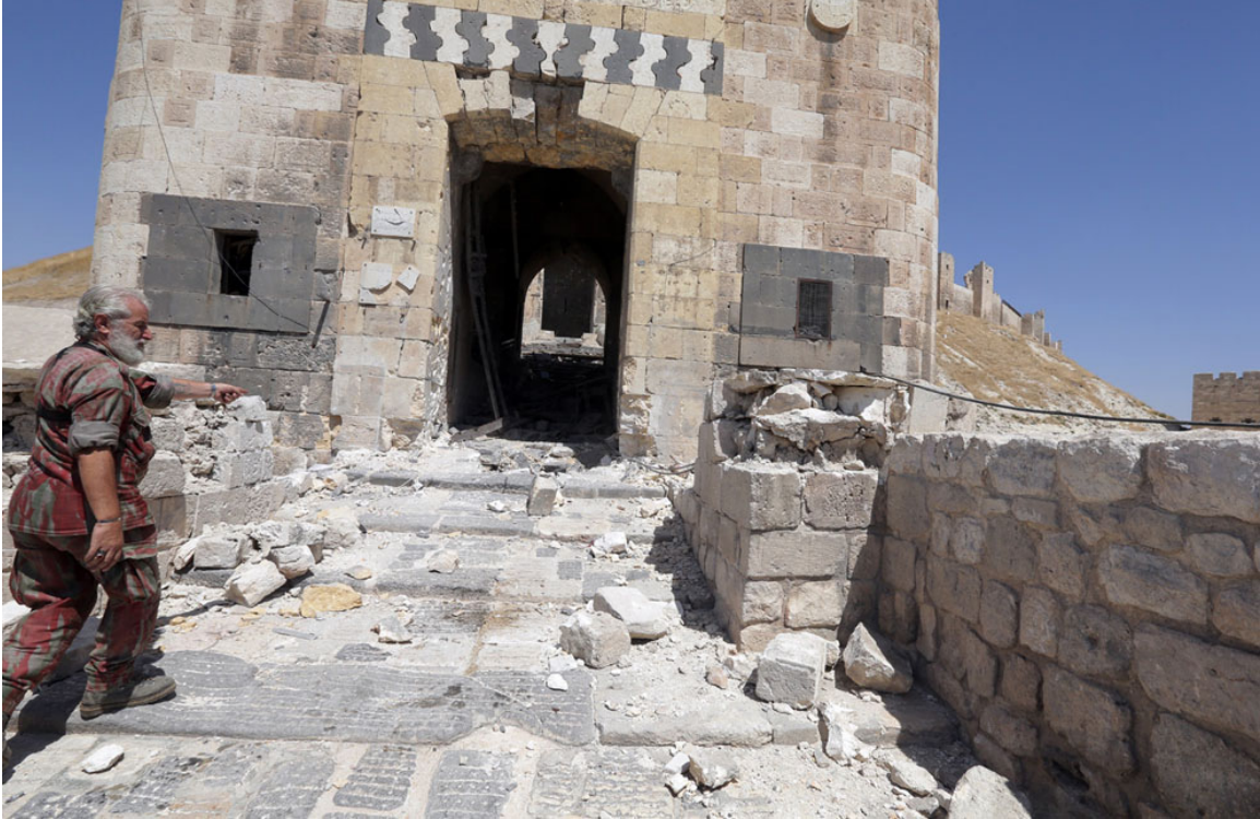
Image showing damage to the Citadel of Aleppo (APSA)
