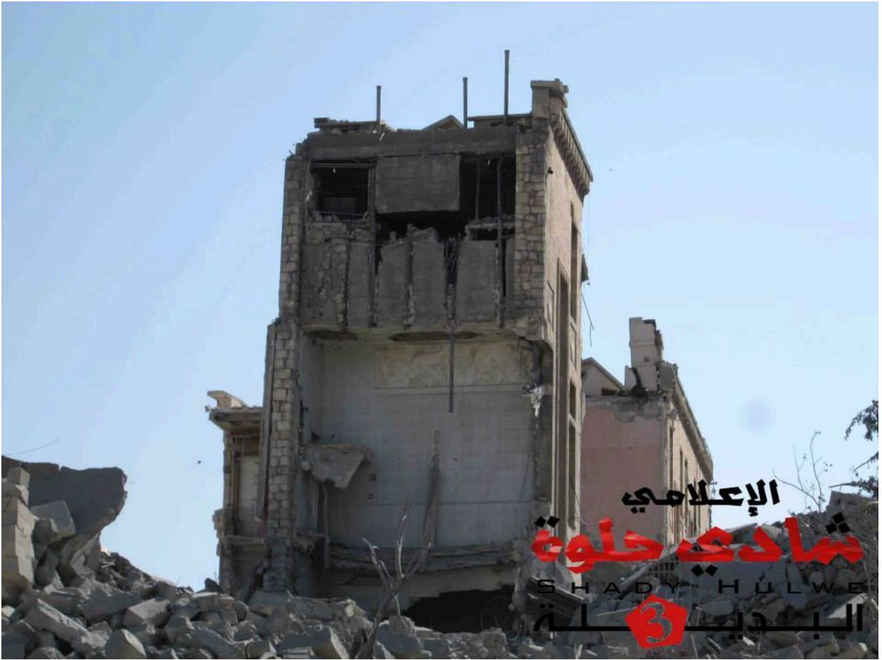
The remains of the Serail in the UNESCO World Heritage Site Old City of Aleppo following the two tunnel bombing of July 29 and two tunnel bombings on September 2, 2014. The neighboring Hammam Yalbougha was also reportedly damaged in the blasts (Shady Hulwe).
