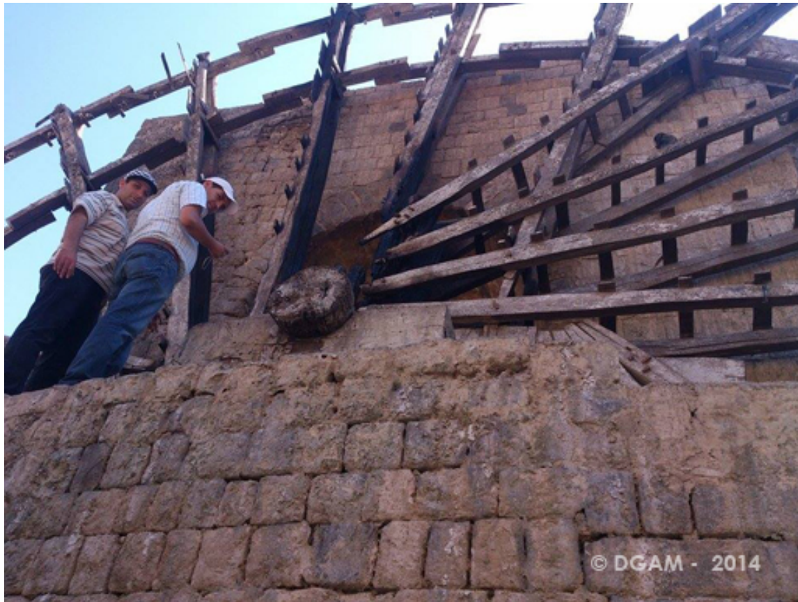
Fire damage to the Noria al-J'berihe, Hama (DGAM).
