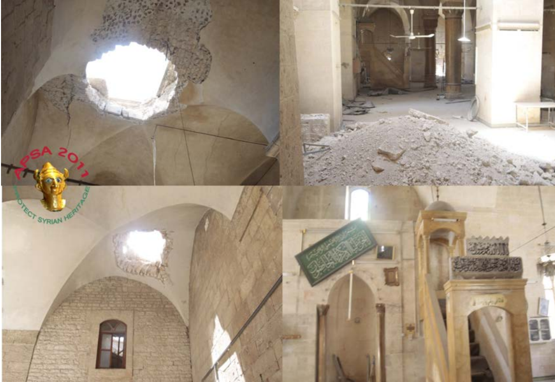
Damage to the al-Otrush Mosque (APSA).
