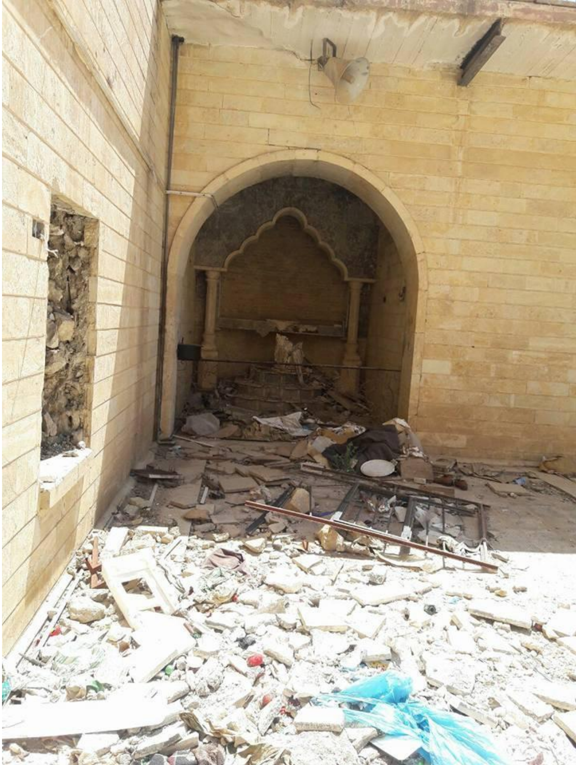
Damage and evidence of intentional destruction seen to Mar Gorgis Monastery (Shlama Foundation; May 9, 2017)
