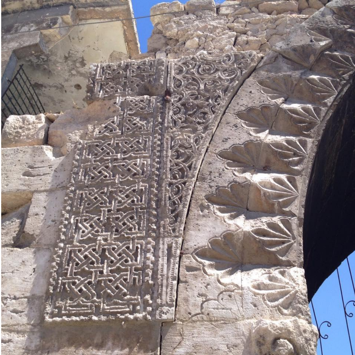
Damage to the facade of Khan Uch Khan (Private Facebook Account; May 21, 2017)
