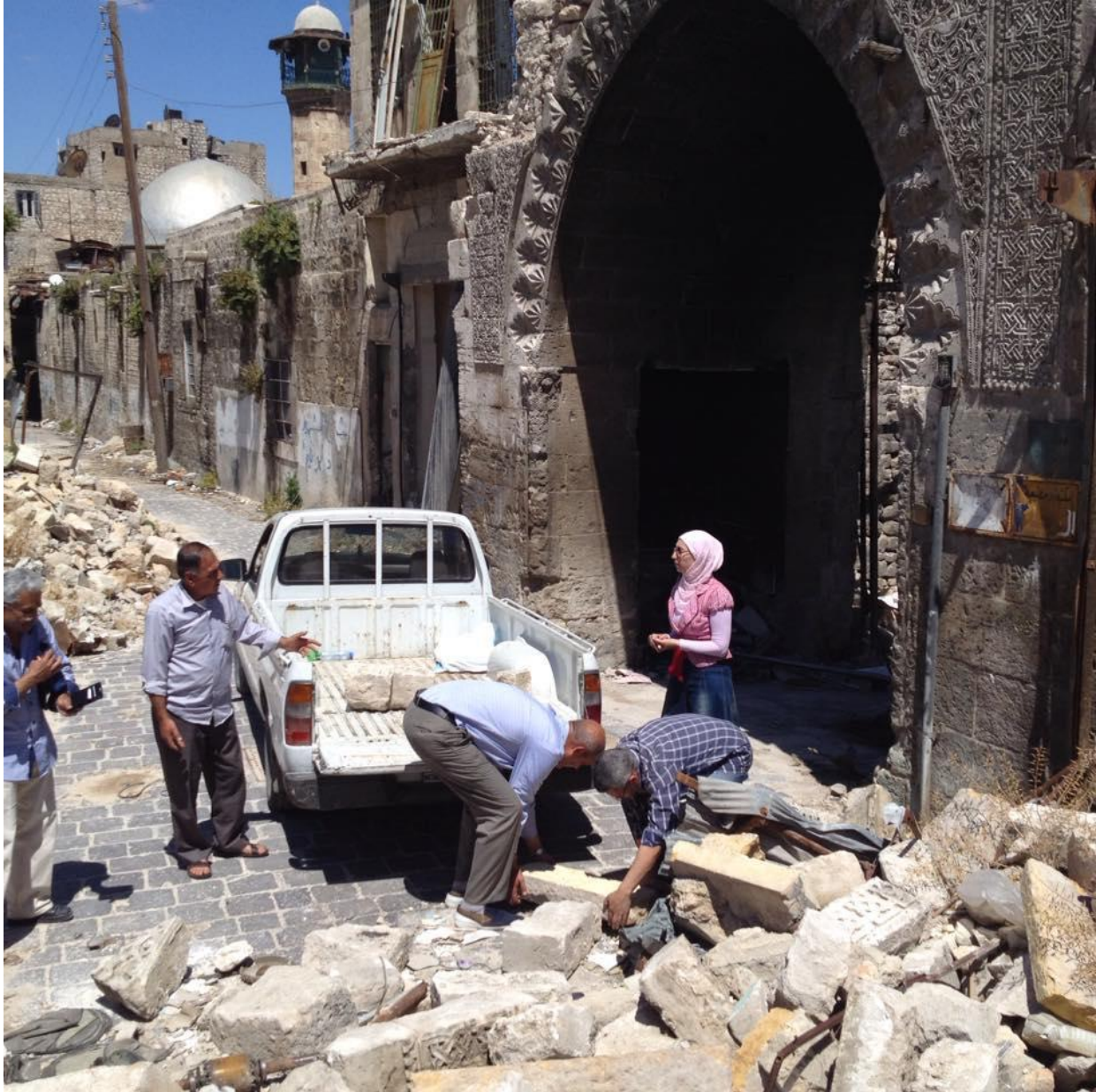
Engineers picking up part of the facade that has fallen from gate (Private Facebook Account; May 21, 2017)
