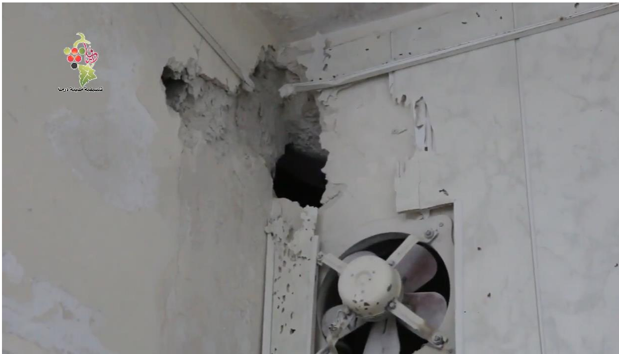
Shelling damage to Hothaifa bin al-Yaman Mosque (SNHR; May 17, 2017)
