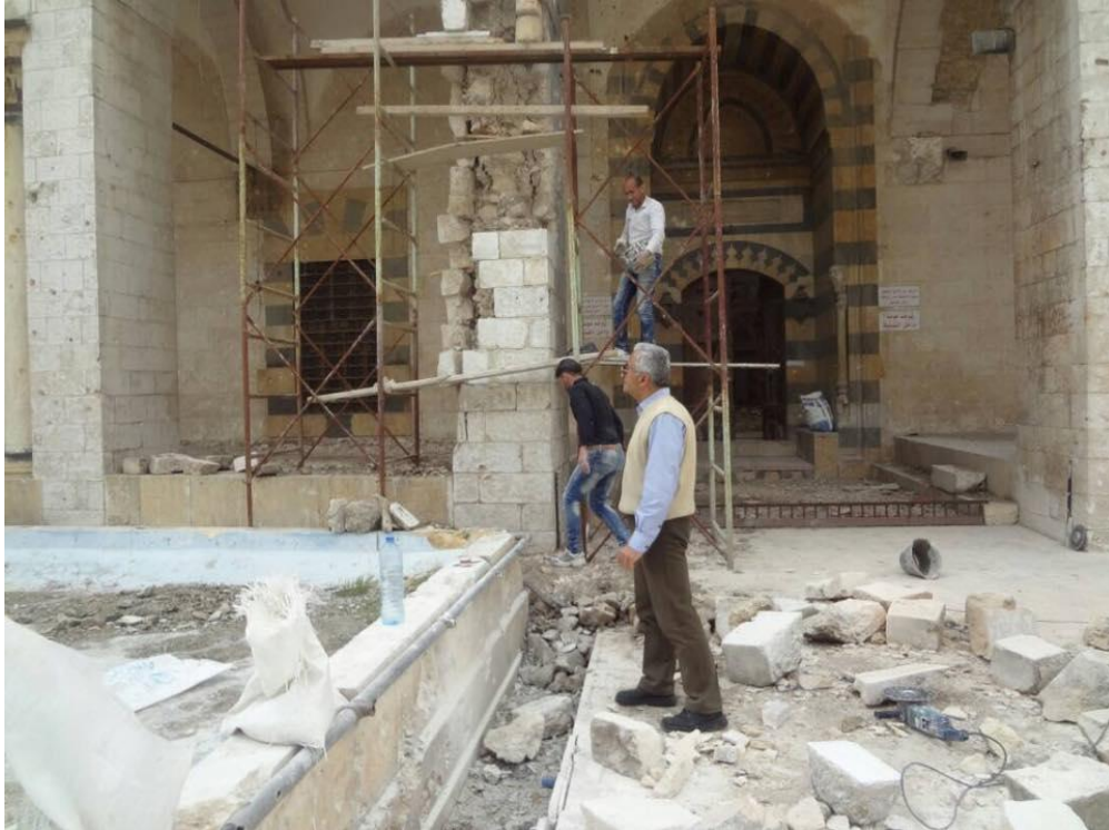
Scaffolding supporting a column at the entrance to the mosque (Private Facebook Account; April 22, 2017)
