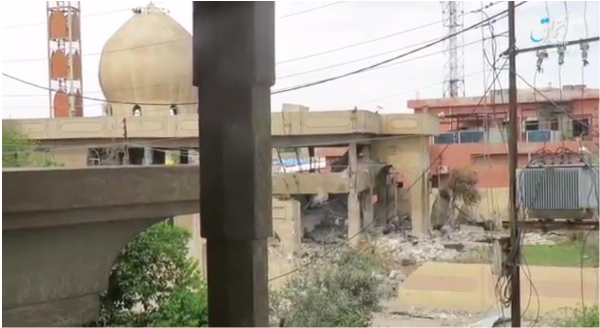
Video still showing severe damage to al-Mufti Mosque (Amaq News Agency; May 18, 2017)
