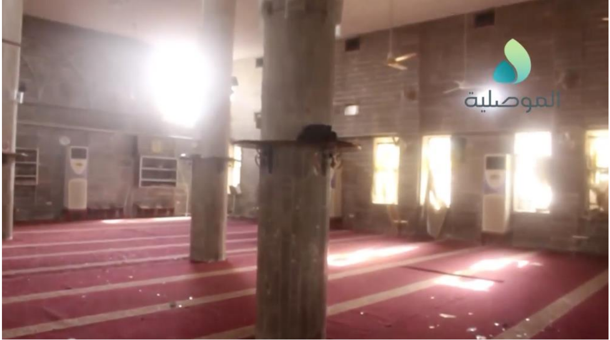
Video still of damage to Yehia al-Talib Mosque (al-Mosuliya Channel; May 19, 2017)
