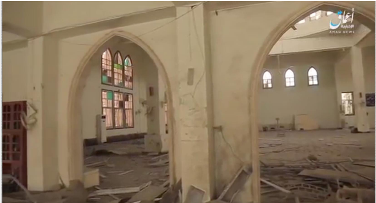
Video still showing damage to interior of the mosque with slight crack in wall, rubble on floor, and missing window panes (Amaq News Agency; May 28, 2017)
