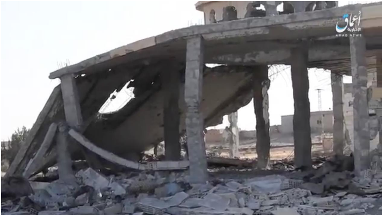
Video still of the destroyed Hamada al-Al'ouwi Mosque (Amaq News Agency; May 8, 2017)
