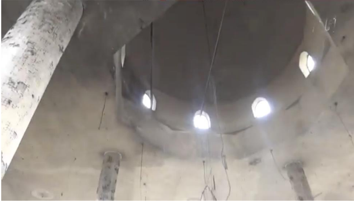
Video still of extensive damage to al-Mufti Mosque (Amaq News Agency; May 1, 2017)
