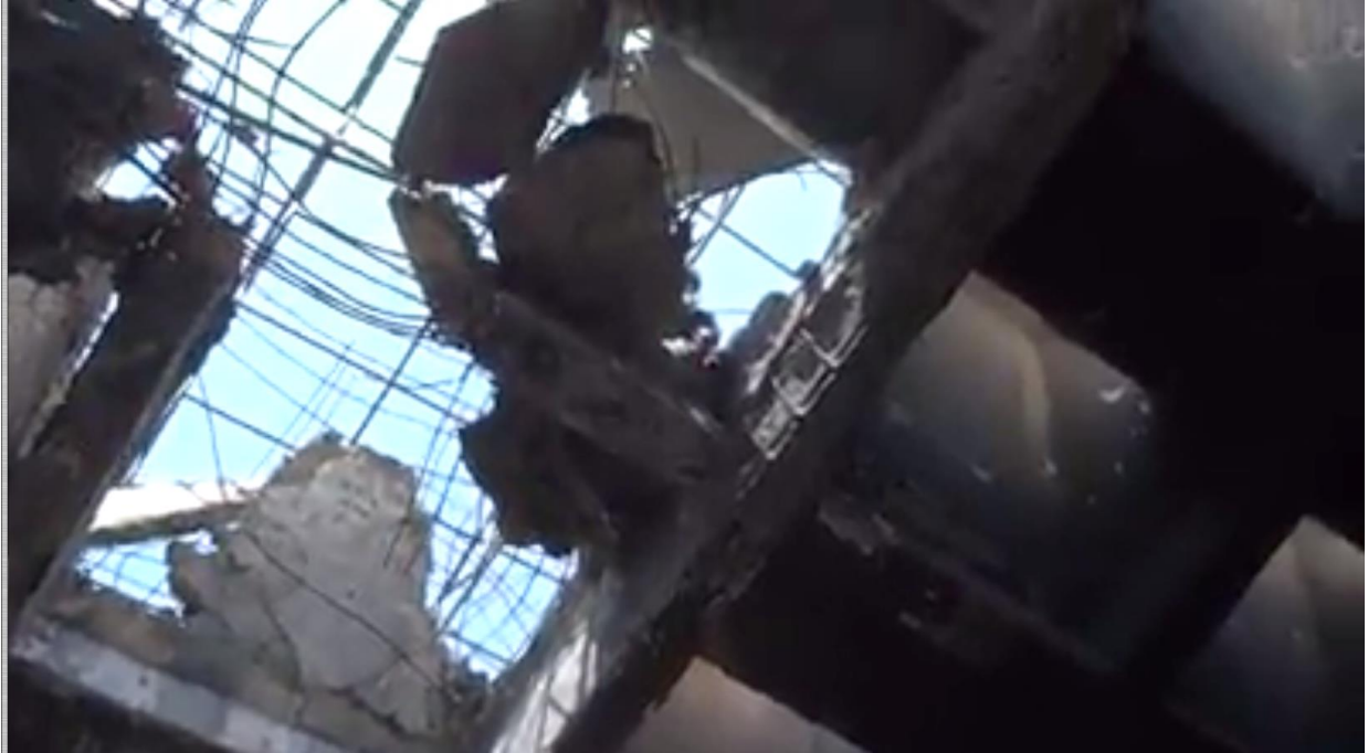
Video still of missing portion of roof in Mosul University Library (Mosul Eye; May 16, 2017)
