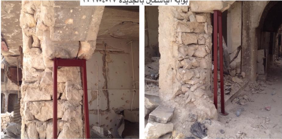
Bawabat al-Yasmin after structural support was placed under the arch (Private Facebook Account; April 27, 2017)
