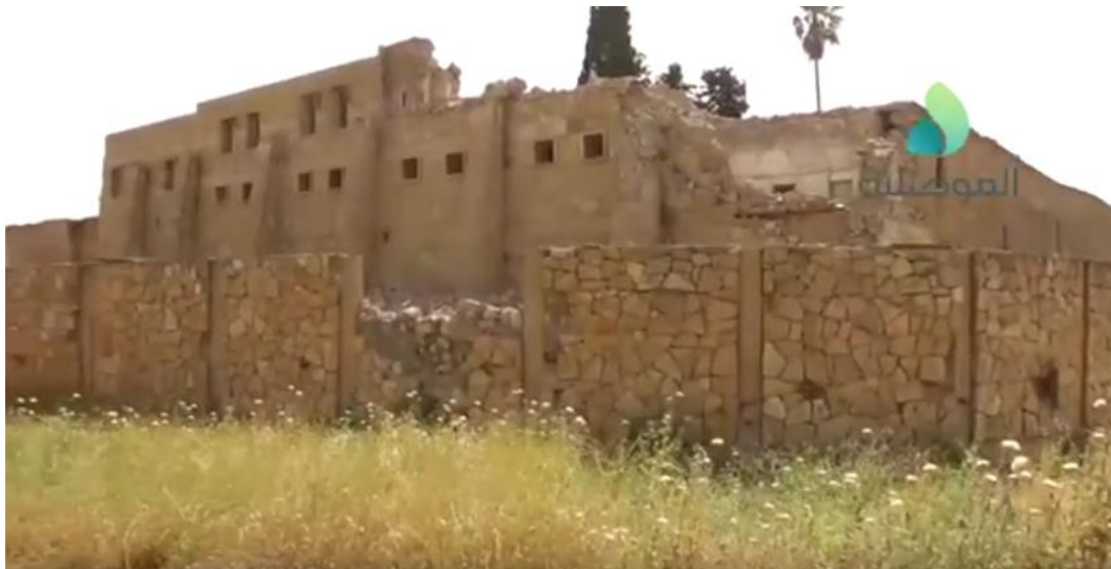
Video still of damage to northeastern corner of Mar Mikhael Monastery (al-Mosuliya; May 16, 2017)
