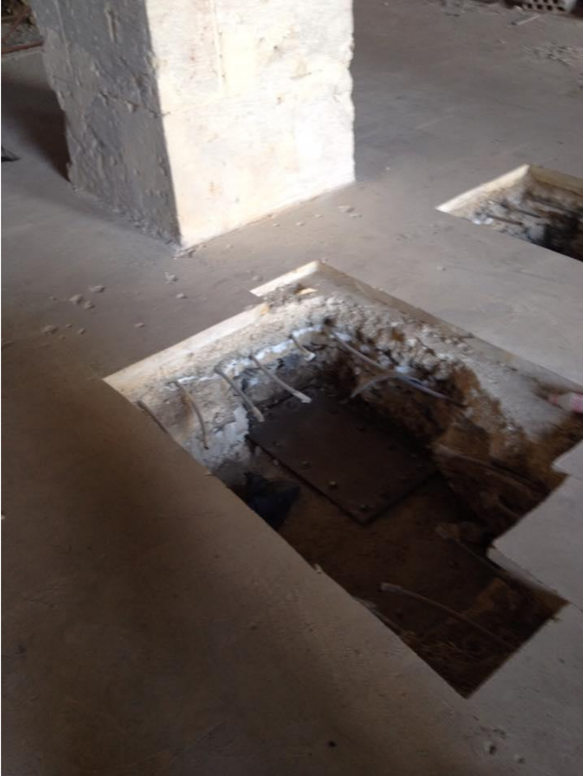
Detail of the hole created for the steel beam (Private Facebook Account; May 1, 2017)
