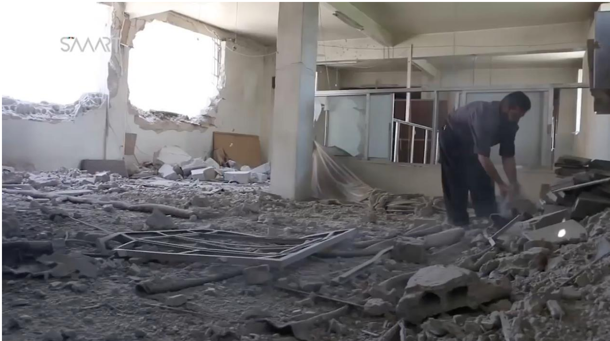
Video still of damage to Hamouriya Grand Mosque (SNHR; May 19, 2017)
