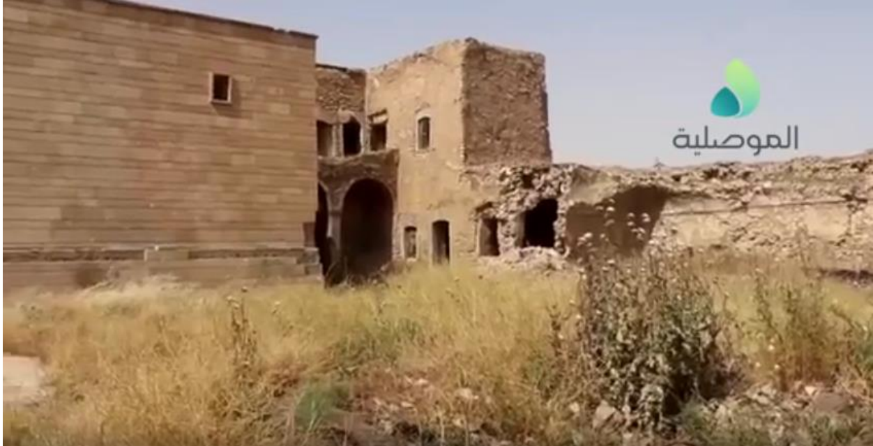
Video still of damage near main entrance to Mar Mikhael Monastery, seen from south (al-Mosuliya; May 16, 2017)
