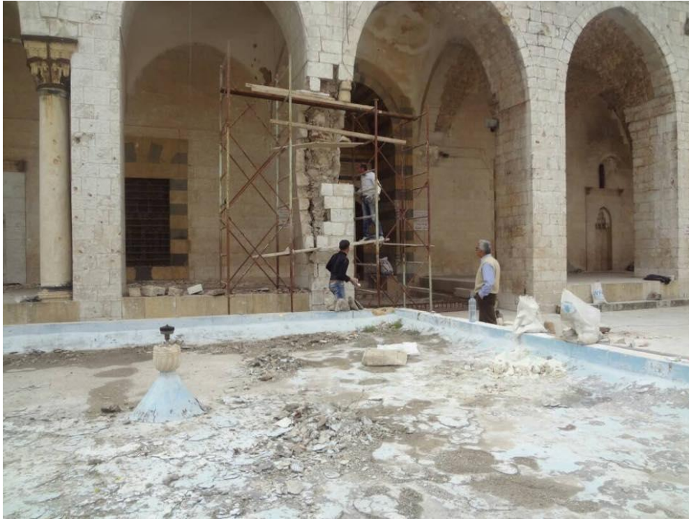
The damaged fountain in the foreground with the stabilized column in the background (Private Facebook Account; April 22, 2017)
