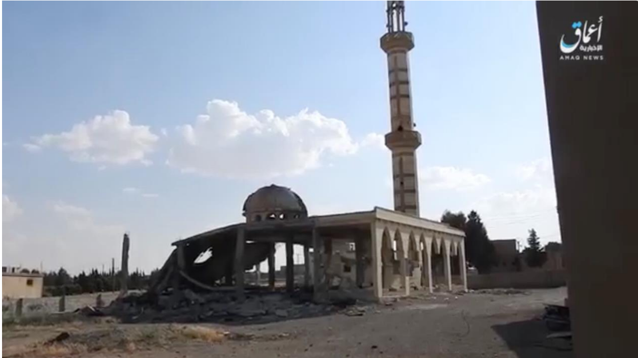
Video still of the destroyed Hamada al-Al'ouwi Mosque (Amaq News Agency; May 8, 2017)
