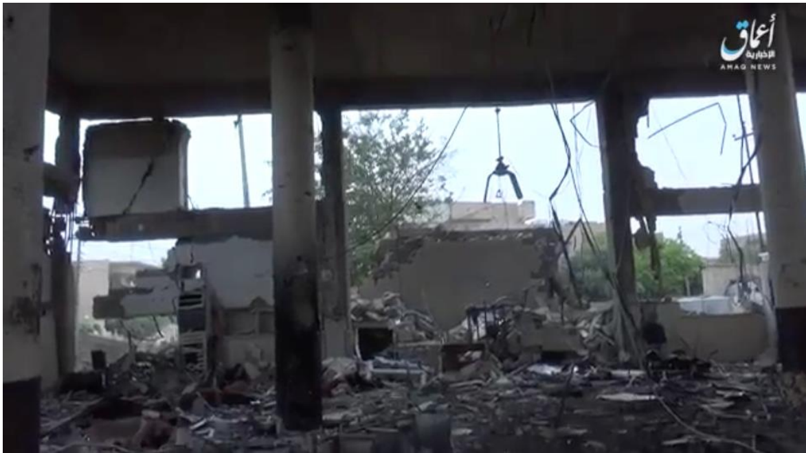
Video still of extensive damage to al-Mufti Mosque (Amaq News Agency; May 1, 2017)
