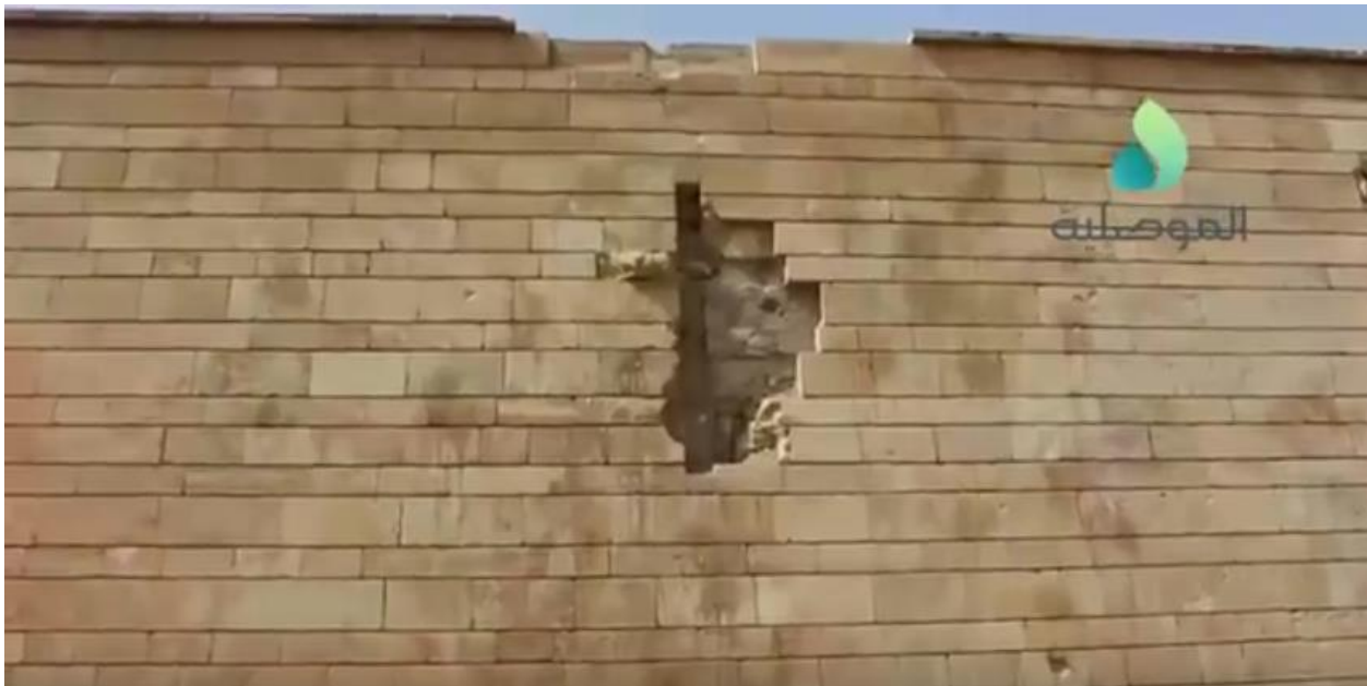
Video still of damage to facade near main entrance to Mar Mikhael Monastery (al-Mosuliya; May 16, 2017)
