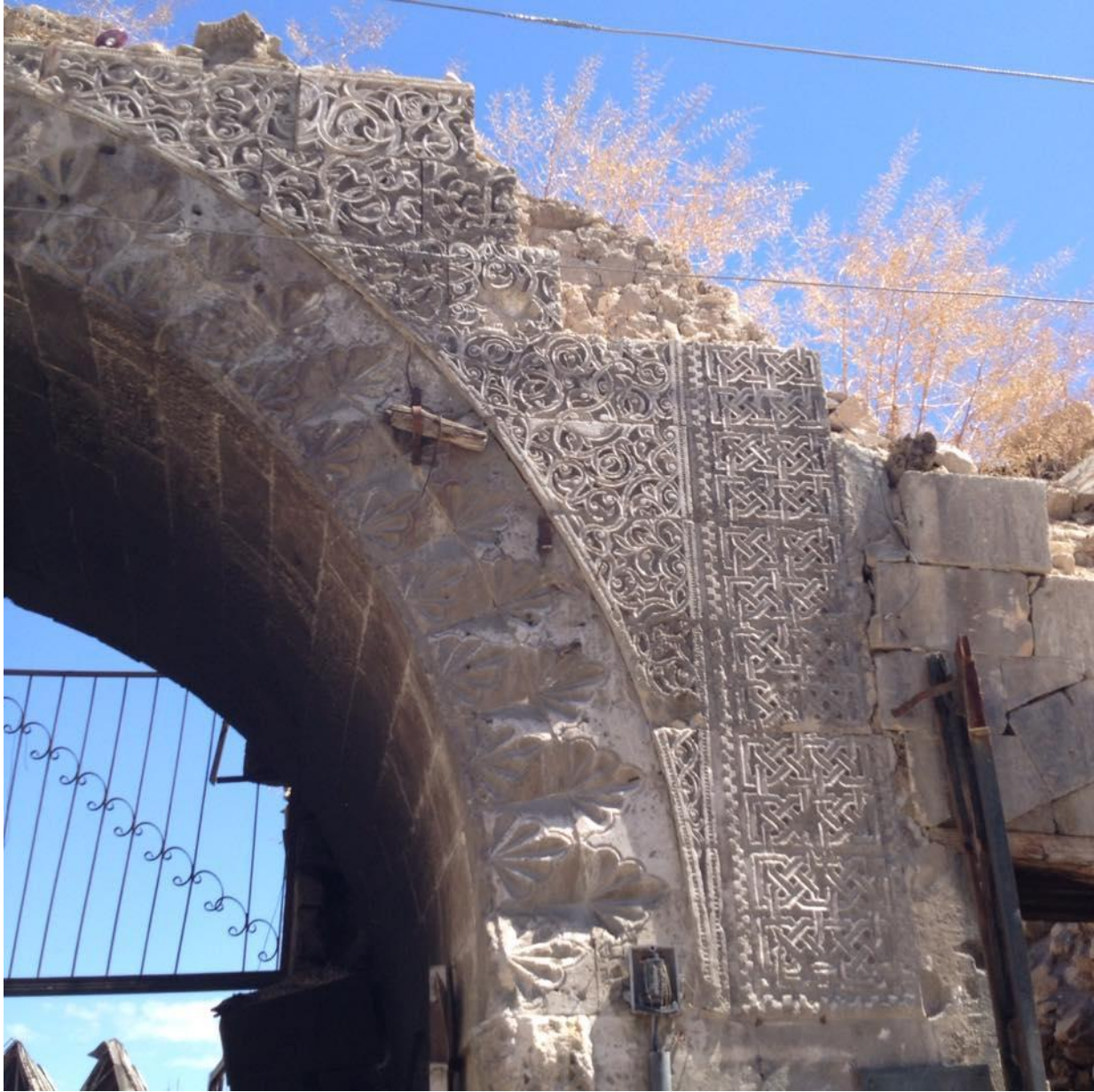
Damage to the facade of Khan Uch Khan (Private Facebook Account; May 21, 2017)
