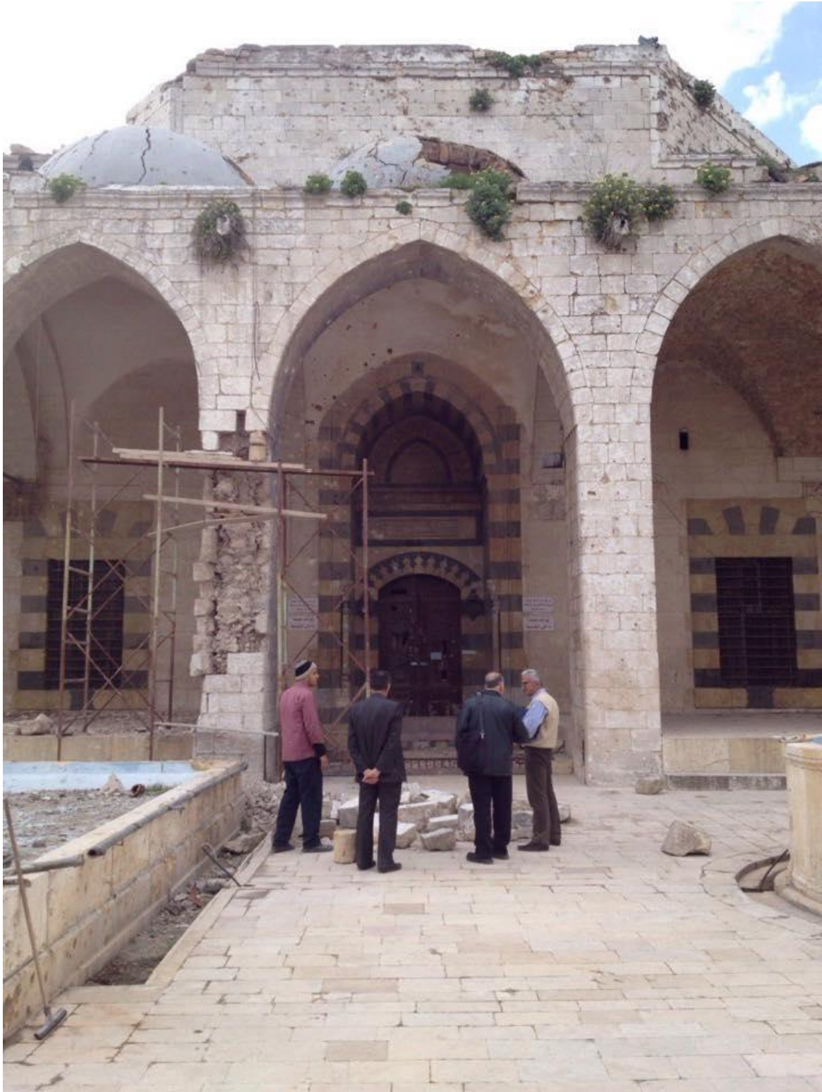
Damage to the mosque, showing location of column before reconstruction (Private Facebook Account; May 31, 2017)
