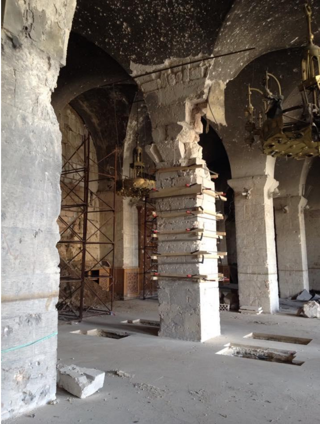
Structural support for the column as well as four holes dug for steel beams to help reinforce the area around the damaged column (Private Facebook Account; May 1, 2017)
