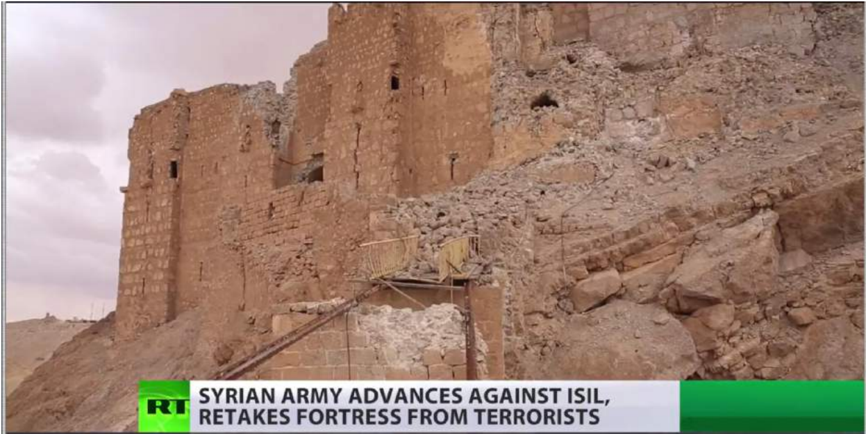
Video still of damage to the front of the Citadel (Ruptly TV; March 1, 2017)
