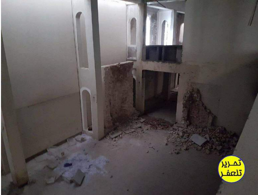
Damage to interior of the Mosul Museum (Personal Twitter Account; March 10, 2017)
