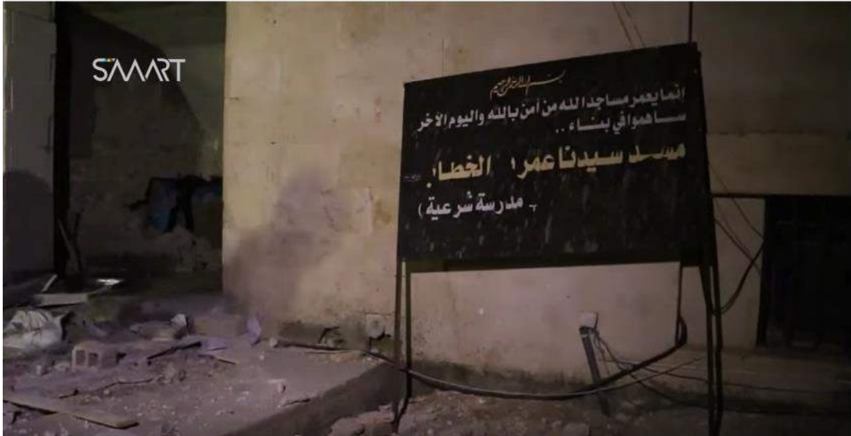
Damage seen to the mosque compound (SMART News Agency; March 16, 2017)
