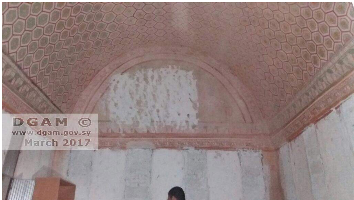
Blocking and plaster over the entrances to the tombs and plaster over part of a painting (DGAM; March 6, 2017)
