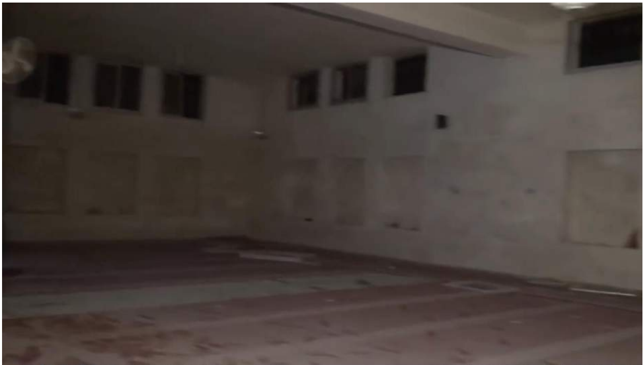
Video still of the moderately damaged musalla of the mosque compound, the room located above has collapsed (Moaz al-Shami; March 16, 2017)
