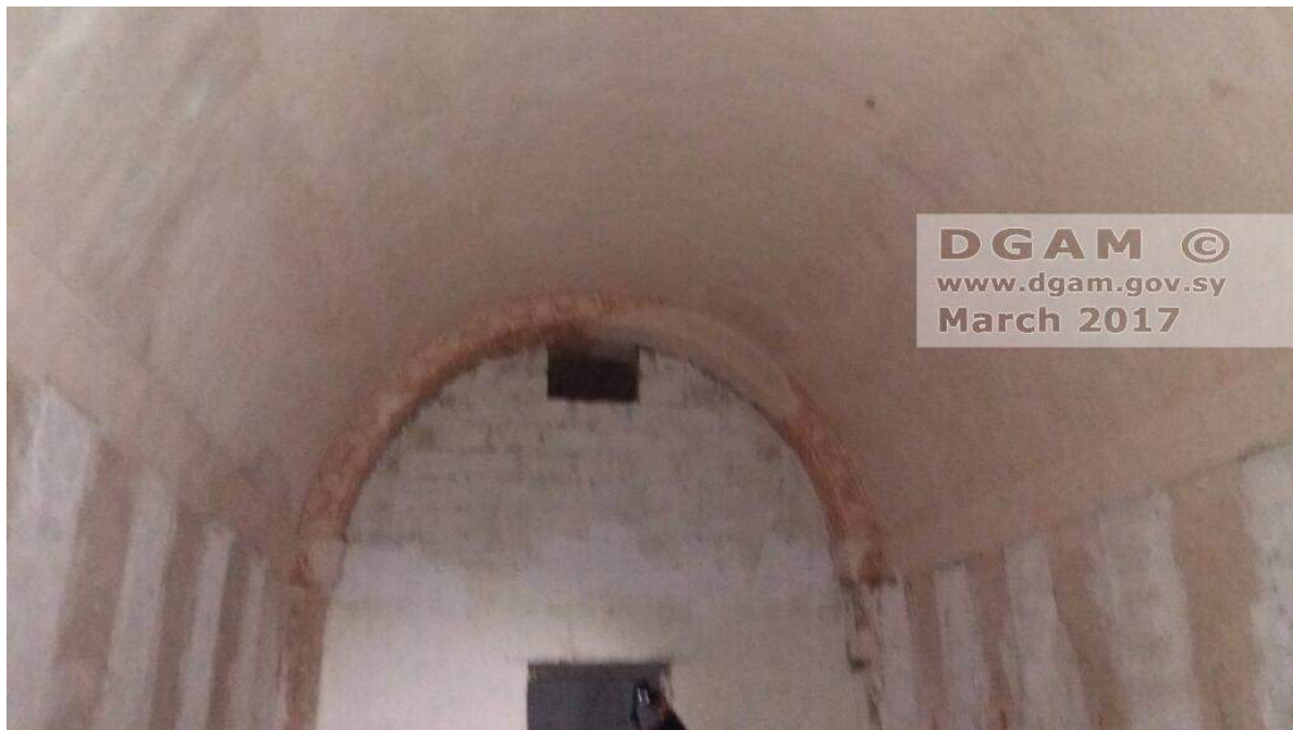
Blocking and plaster over the entrances to the tombs, and restoration of the end of the Hypogeum (DGAM; March 6, 2017)
