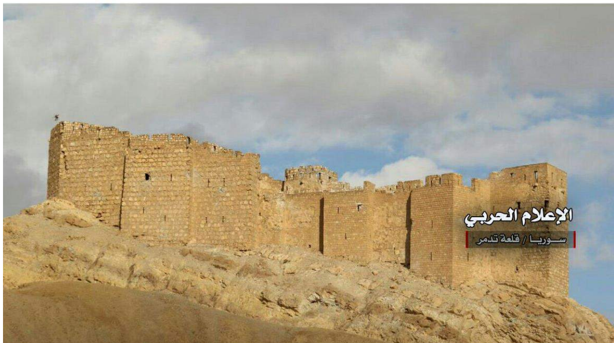
Damage to the back of the Citadel (Private Twitter Account: March 2, 2017)
