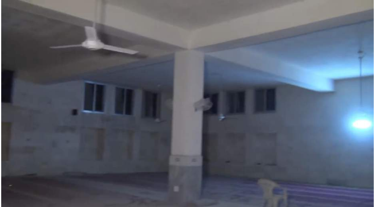
Video still of the moderately damaged musalla of the mosque compound, the room located above has collapsed (Moaz al-Shami; March 16, 2017)
