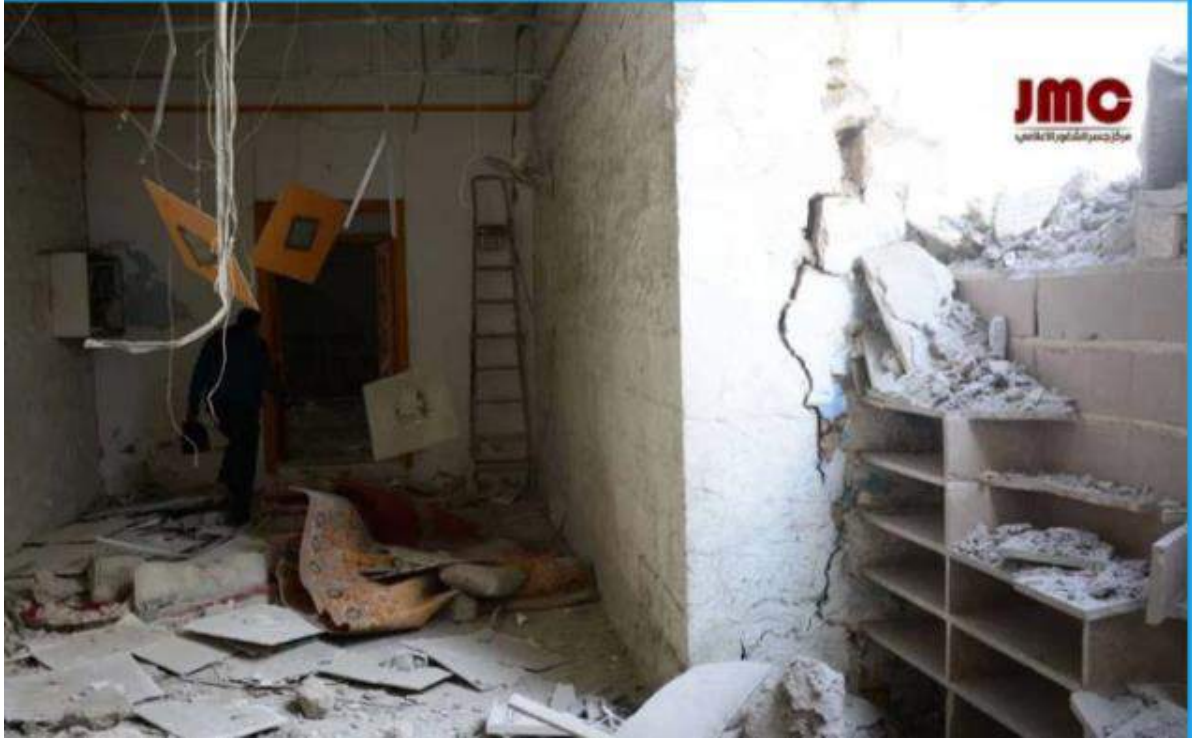
Damage to the interior of the mosque (SNHR; April 13, 2017)
