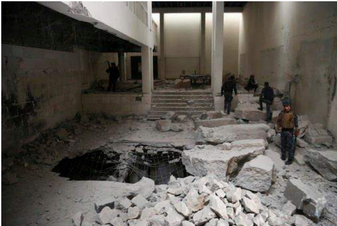
Damage to the interior of the Mosul Museum (Khalid Mohammed/AP; March 8, 2017)
