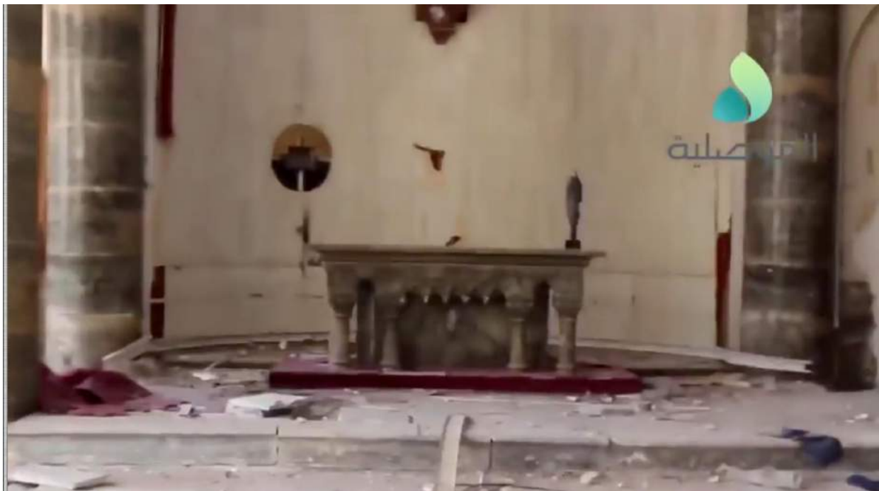
Video still of damage to the altar of Umm al-Mauna Church (al-Mosuliya; March 11, 2017)
