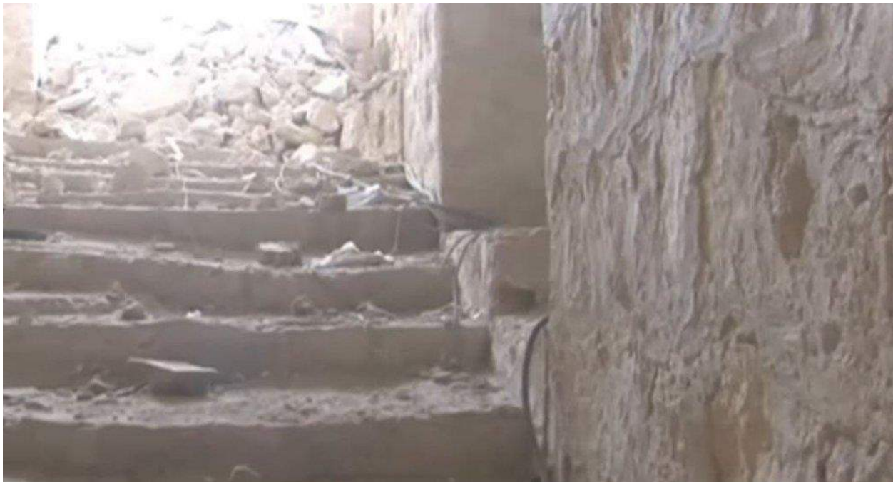
Video still of damage to the stairs inside the Citadel (Ruptly TV; March 1, 2017)
