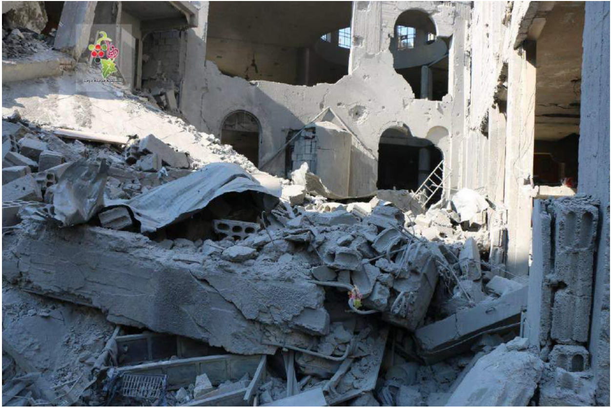
Damage to exterior of mosque (SNHR; April 13, 2017)
