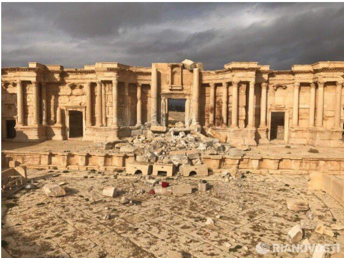
Damage to the front and stage of the theater (Private Twitter Account; March 2, 2017)
