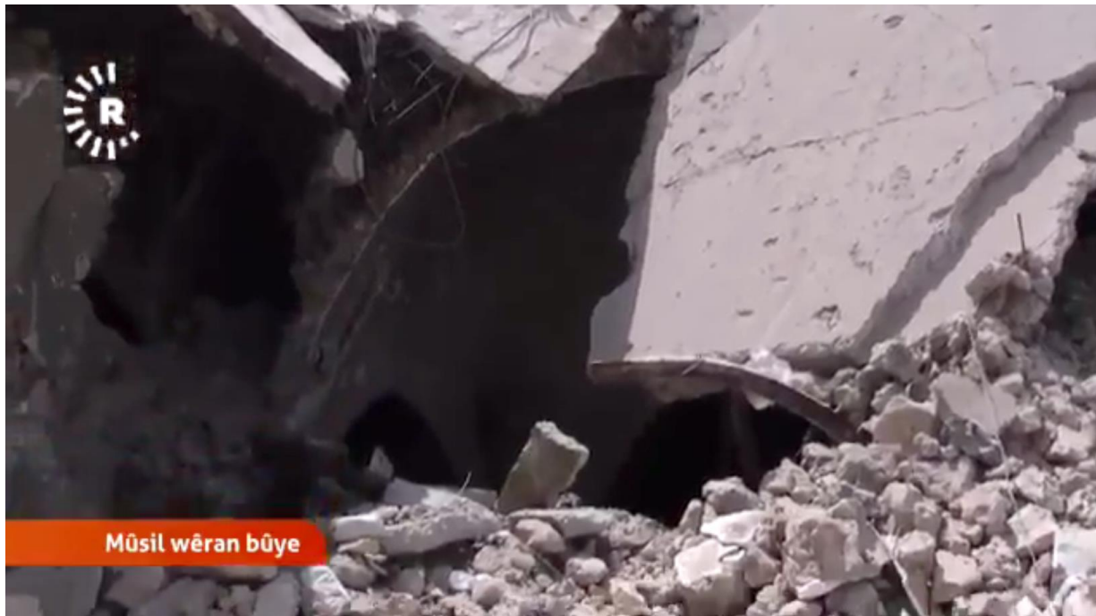
Video still of damage to al-Aghwat Mosque (Rudaw; July 10, 2017)
