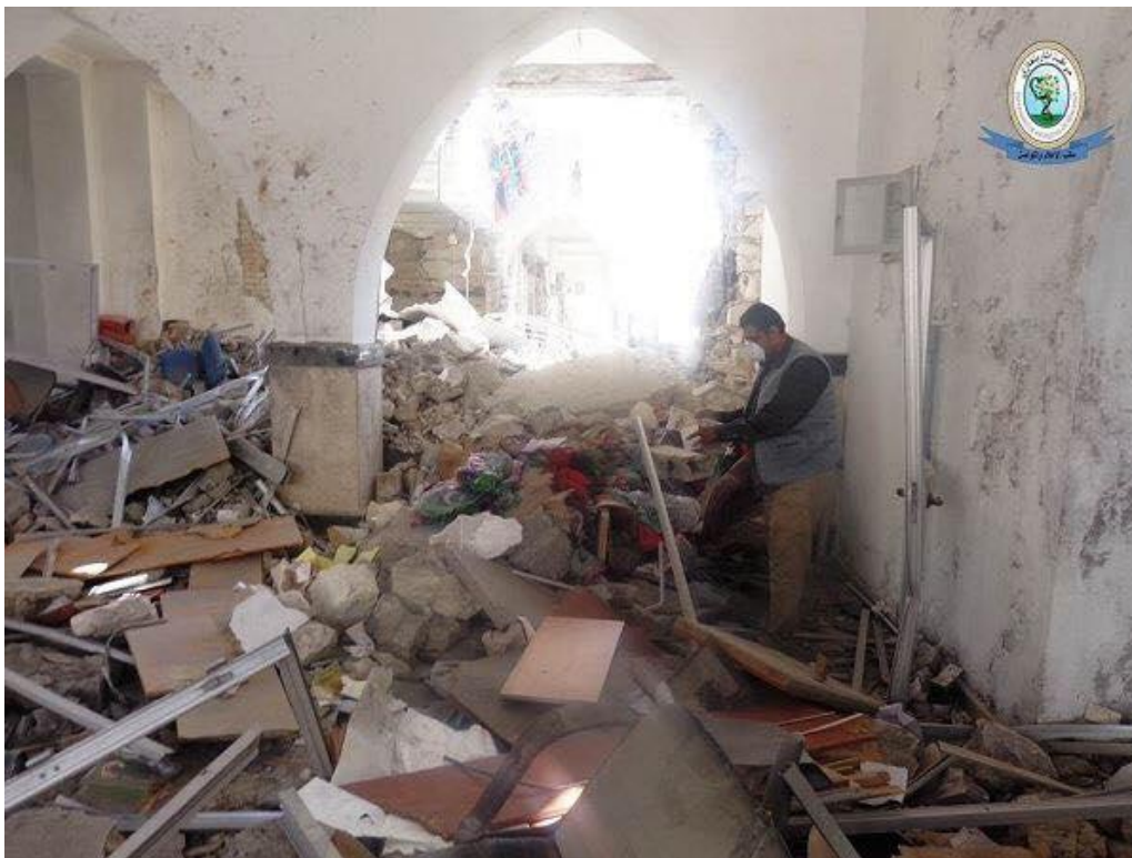
Additional view of the damage to the DoA Benghazi headquarters (Abdel Hafid al-Massalati; July 20, 2017)
