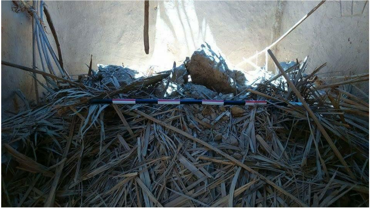
Interior view of the rubble of the collapsed dome (Meloud Betron; July 20, 2017)
