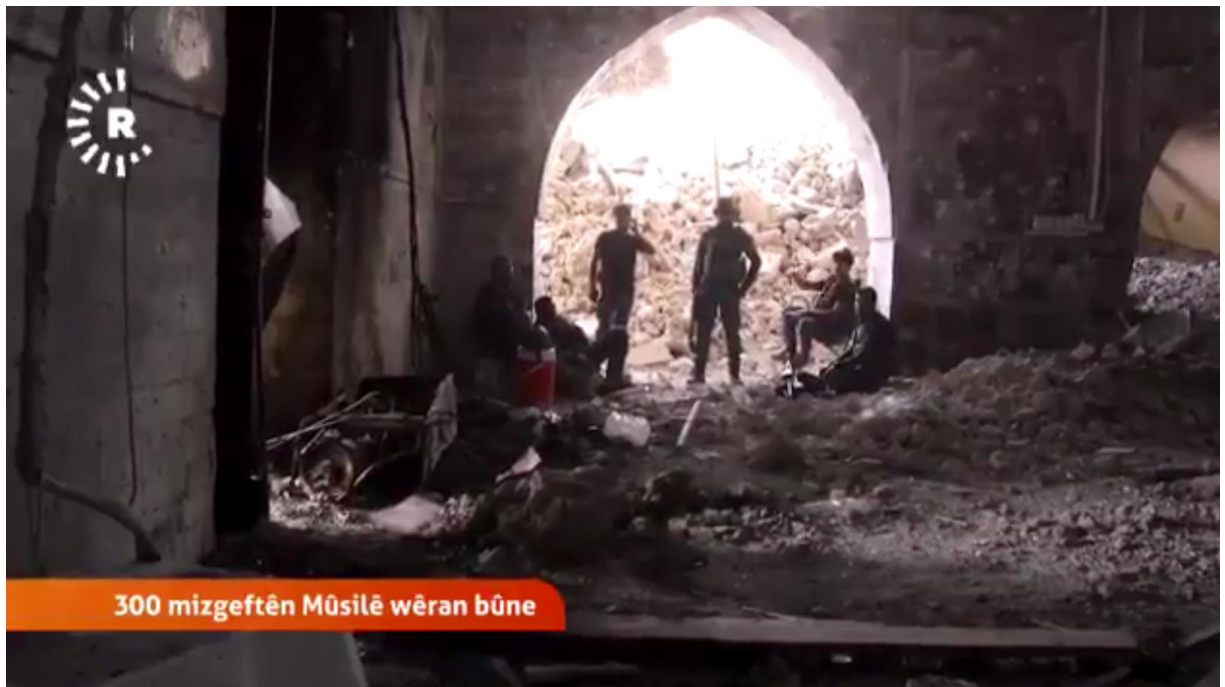
Video still of damage to the interior of al-Aghwat Mosque (Rudaw; July 10, 2017)
