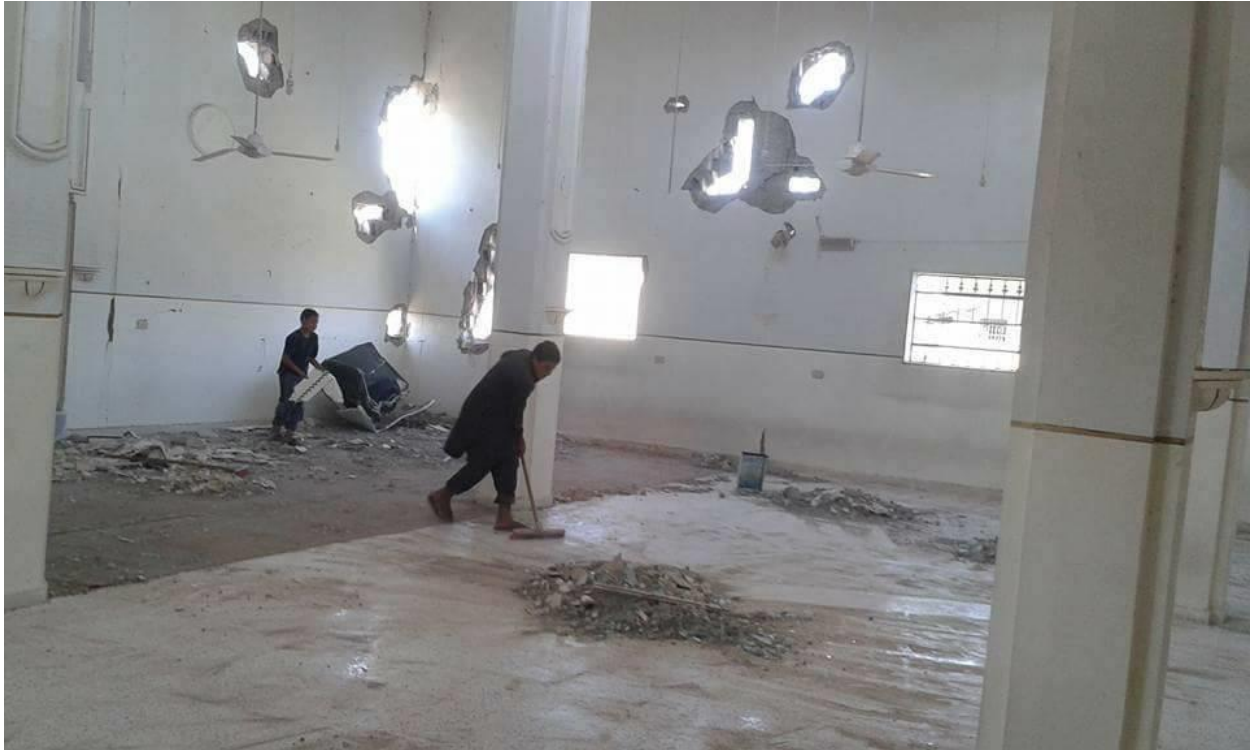
Damage to the walls and contents of the Sa'ad bin Mo'ath Mosque (SNHR; July 24, 2017)
