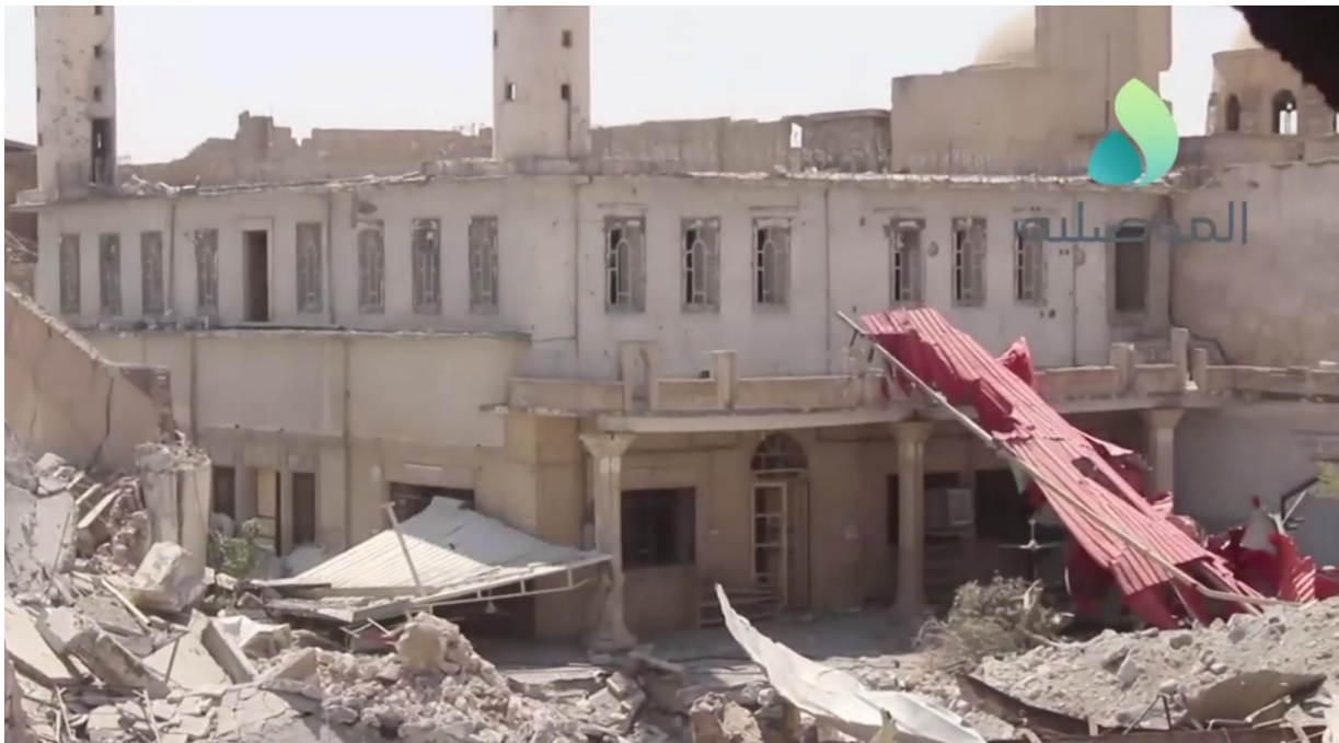
Video still of damage to al-Safar Mosque, the red material seen is part of roofing over the neighborhood to protect people from airstrikes (al-Mosuliya June 29, 2017)
