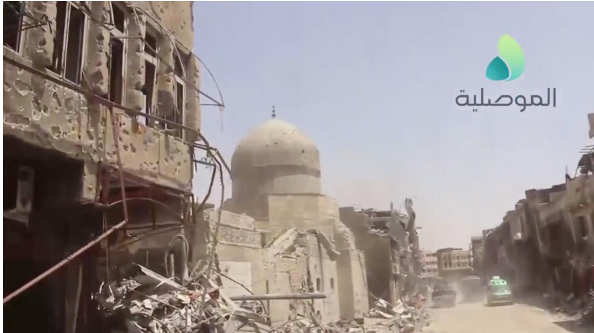
Video still of damage to al-Qataneen Mosque and neighborhood (al-Mosuliya; July 12, 2017)
