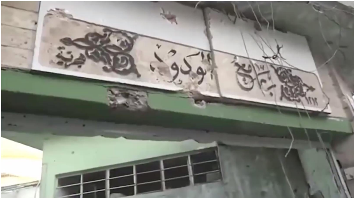
Video still of damage to the exterior of al-Hamdeen Mosque (WK Ahmed; June 23, 2017)
