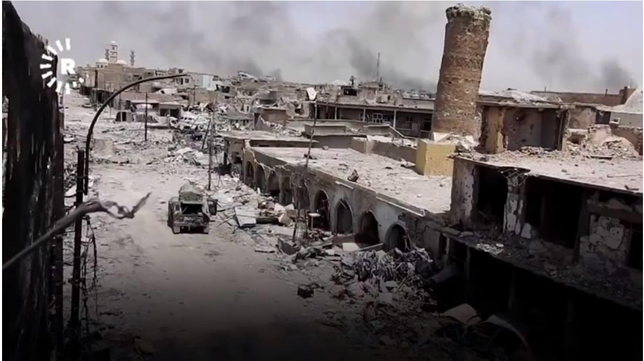
Video still of the Omar al-Aswed Mosque showing damage to the minaret, which is missing its top half and outer facade of building (Rudaw; July 4, 2017)
