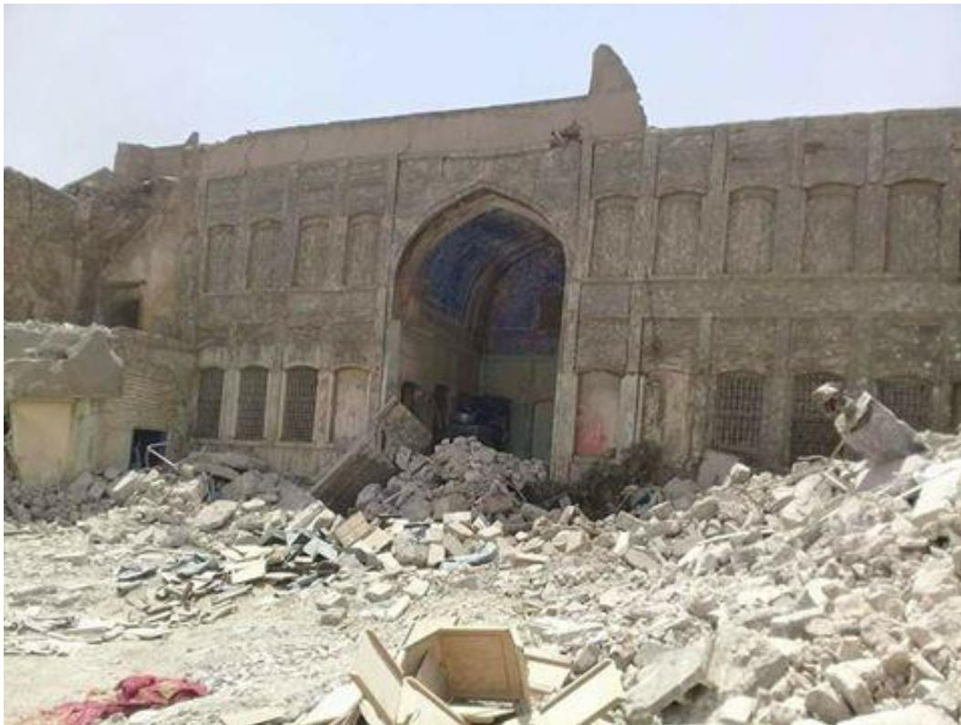
Damage to Dar Thun Hadid with rubble in the courtyard (Private Facebook Account; July 3, 2017)
