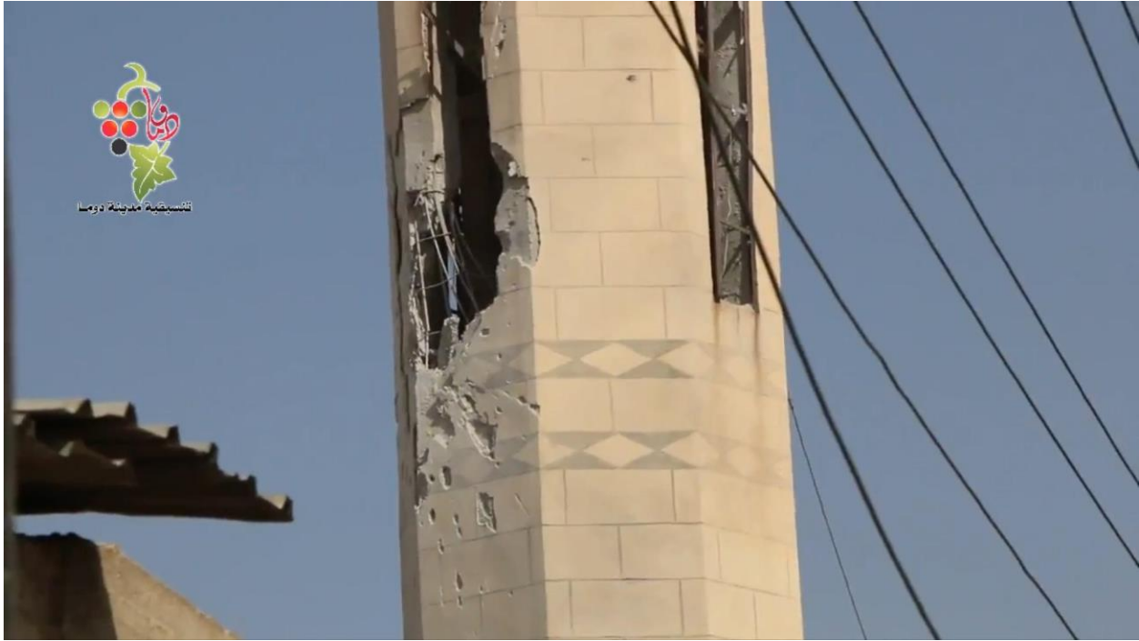
Damage to the minaret of al-Aqoula Mosque (SNHR; July 31, 2017)
