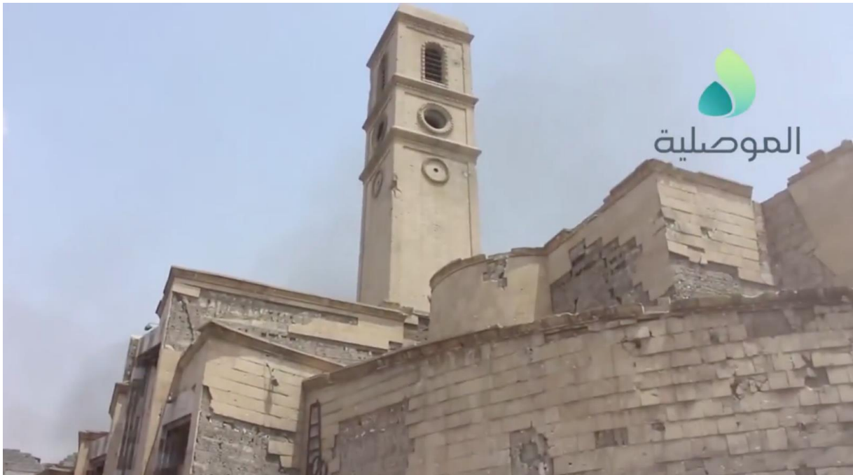
Video still of damage to the northwestern corner of al-Sa'a Church (al-Mosuliya; July 3, 2017)
