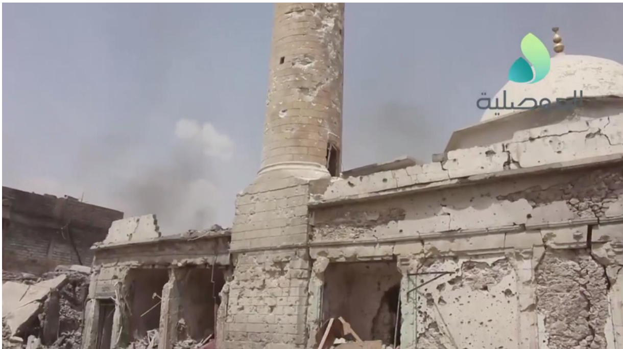
Video still of damage to the western facade of al-Juwayjati Mosque (al-Mosuliya; July 3, 2017)
