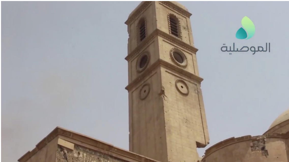
Video still of damage to the clocktower of al-Sa'a Church (al-Mousilya; July 3, 2017)
