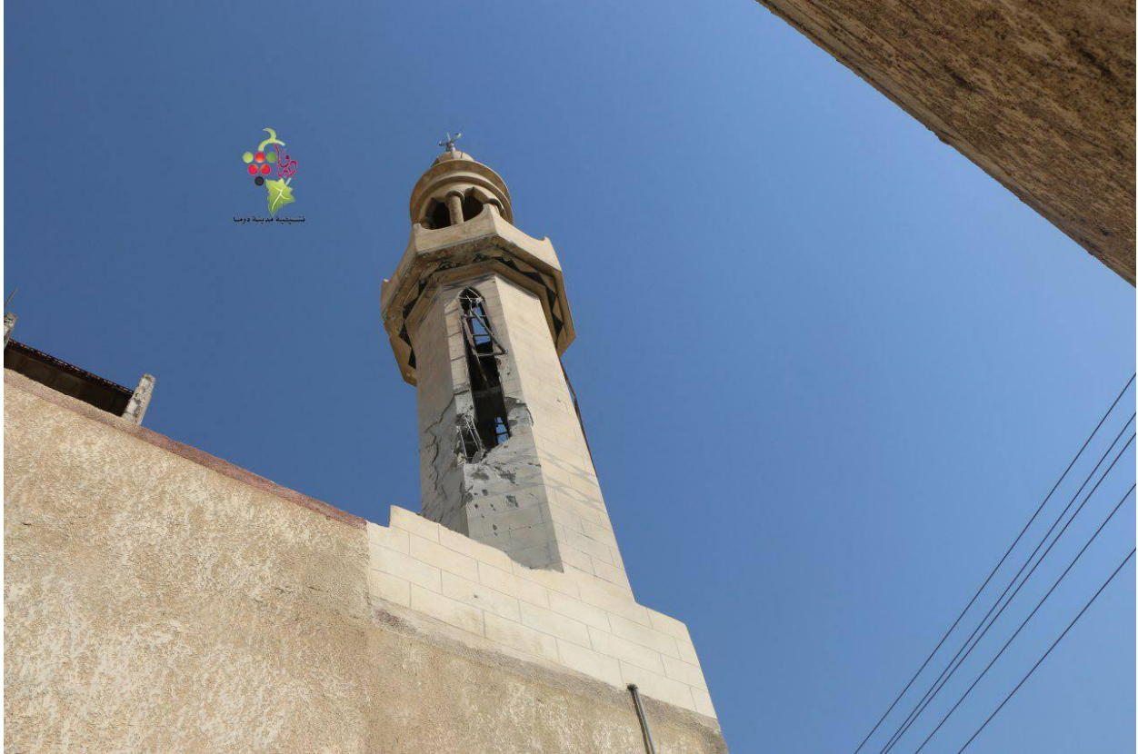
Damage to the minaret of al-Aqoula Mosque (SNHR; July 18, 2017)
