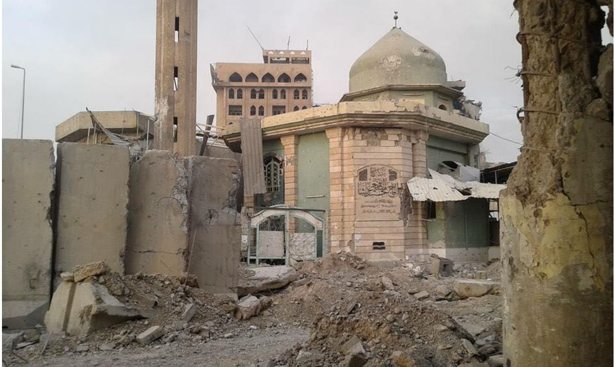
Damage to the al-Pasha Mosque and minaret (Mosul Ateka; July 10, 2017)
