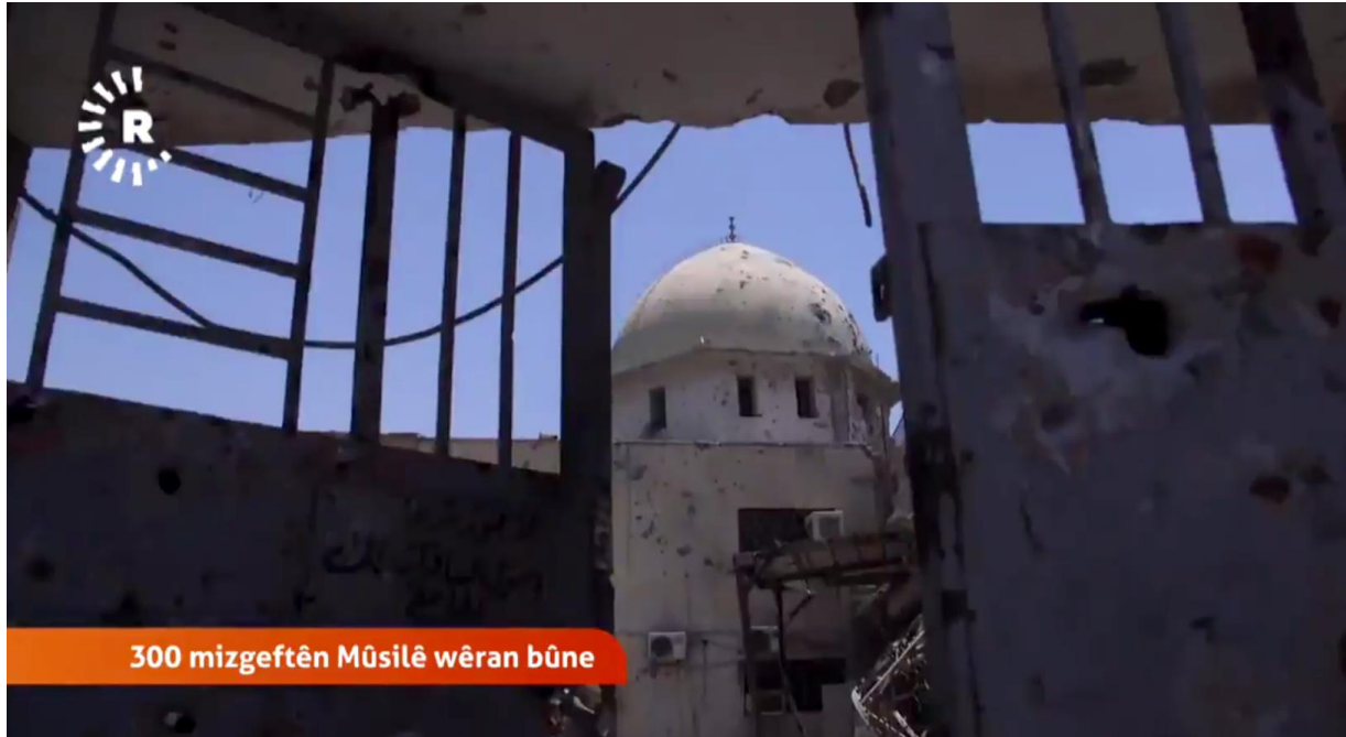
Video still of damage to the interior courtyard and exterior doors of al-Ziwani Mosque (Rudaw; July 10, 2017)
