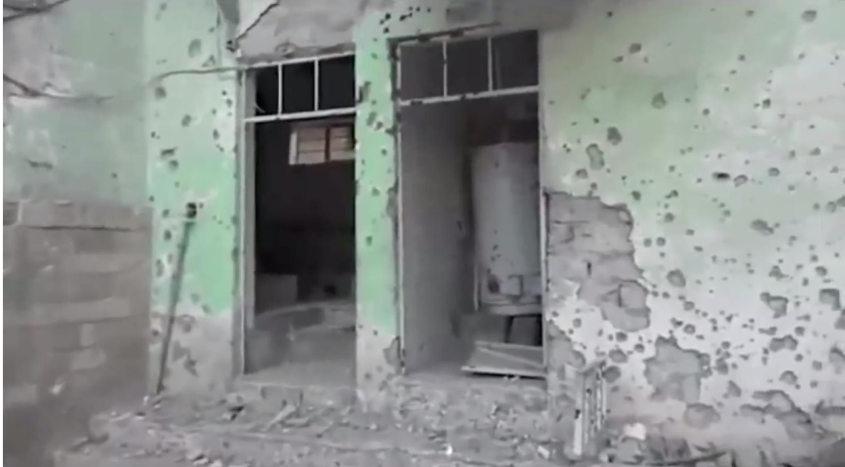
Video still of damage to the courtyard of al-Hamdeen Mosque (WK Ahmed; June 23, 2017)
