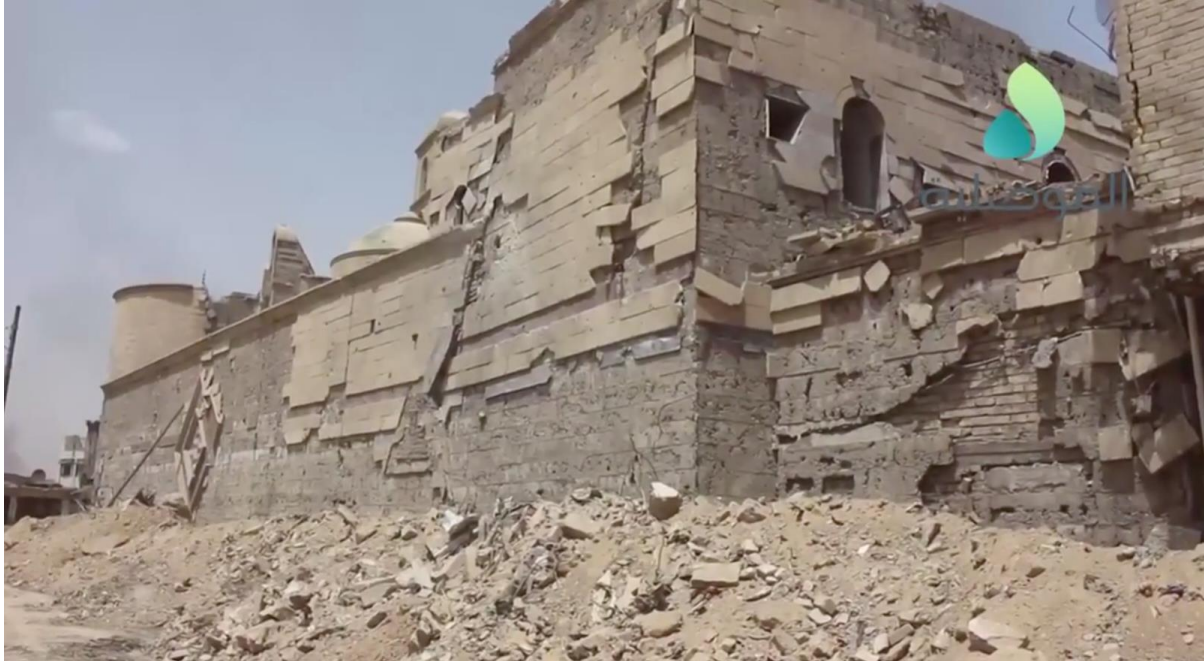
Video still of damage to the western side of al-Sa'a Church (al-Mosuliya; July 3, 2017)
