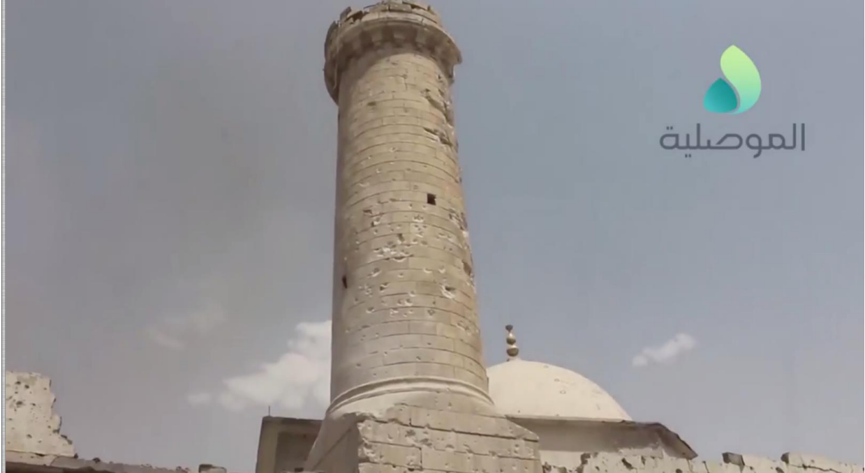
Video still of damage to the minaret of al-Juwayjati Mosque which is missing its top half (al-Mosuliya; July 3, 2017)
