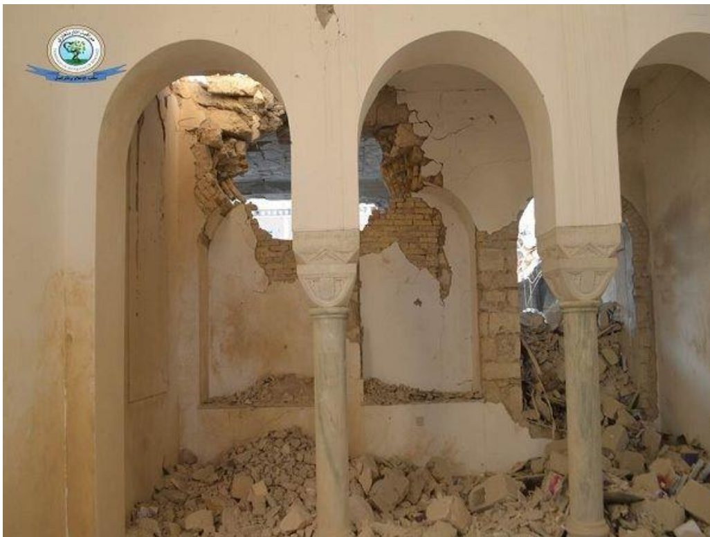
Heavily damaged section of wall (DoA Benghazi; June 28, 2017)
