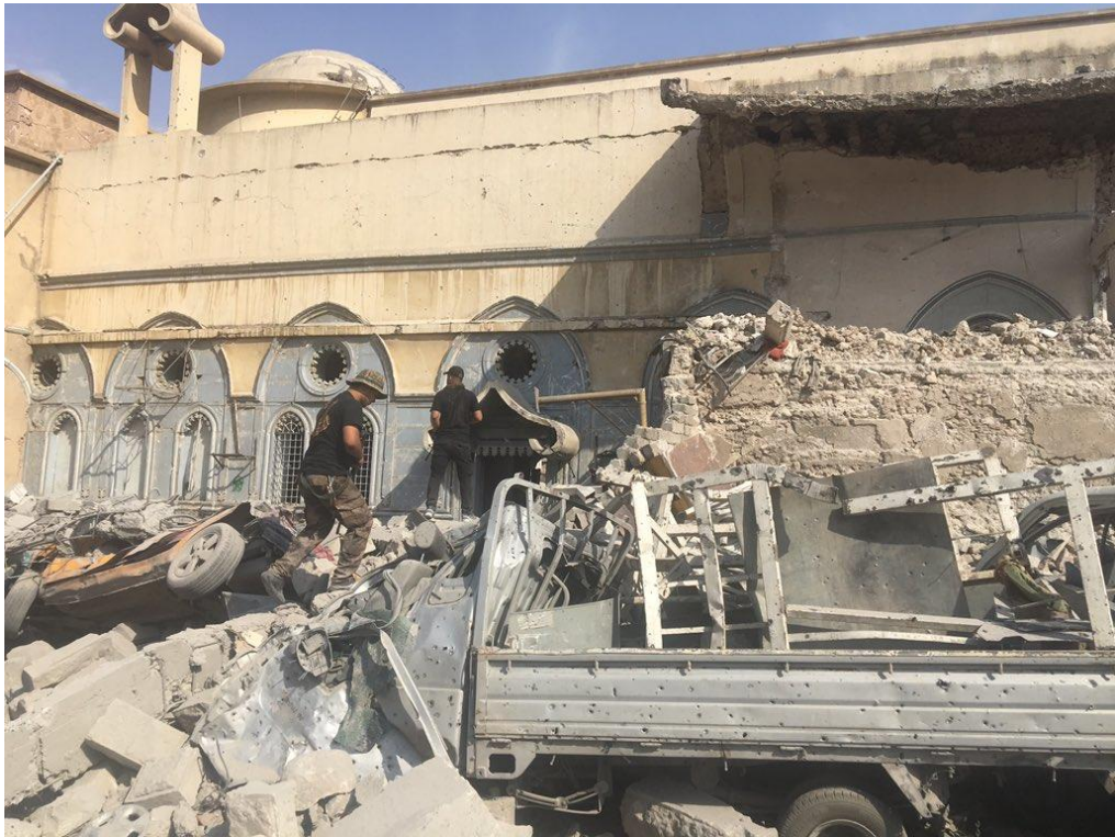
Damage to the exterior of Syriac Orthodox Church (Rukmini Callimachi/NYT; July 11, 2017)
