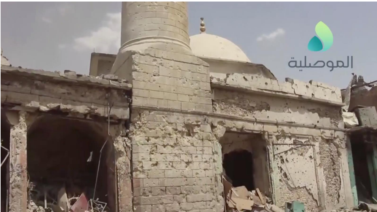
Video still of damage to the western side of al-Juwayjati Mosque (al-Mosuliya; July 3, 2017)
