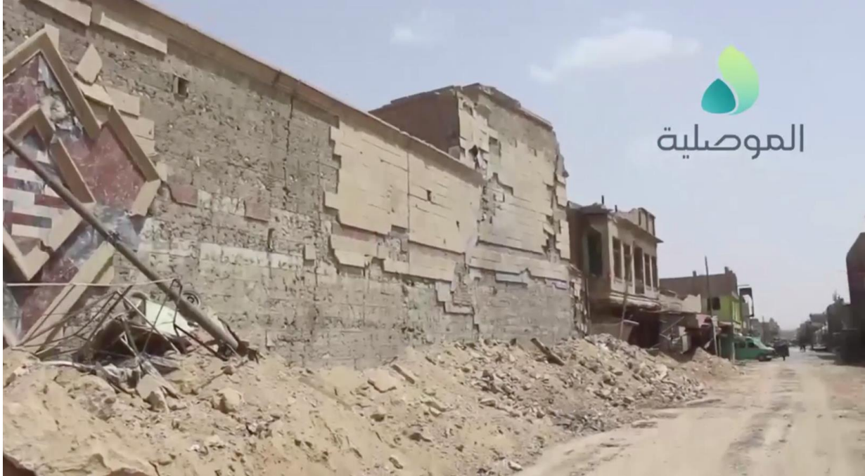
Video still of damage to the western side of al-Sa'a Church (al-Mosuliya; July 3, 2017)
