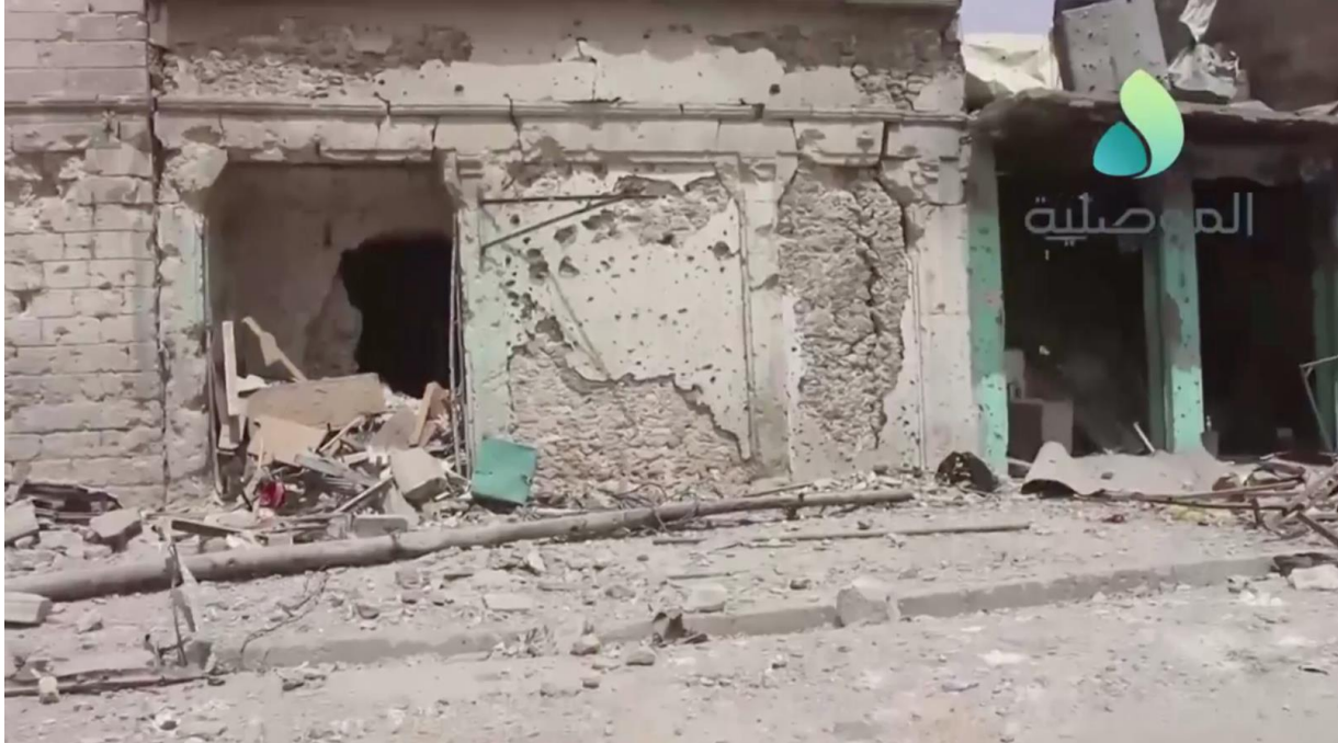
Video still of damage to the western side of al-Juwayjati Mosque (al-Mosuliya; July 3, 2017)
