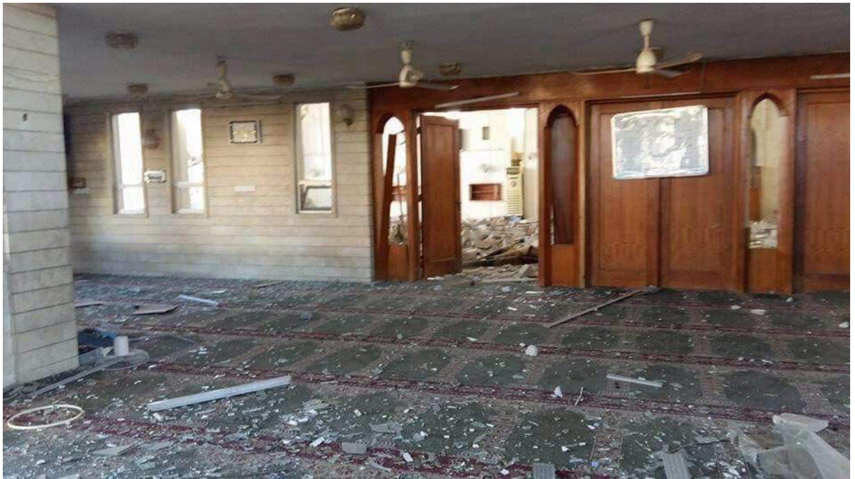
Shattered glass inside the al-Sayegh Mosque (DOAM; January 14, 2017)
