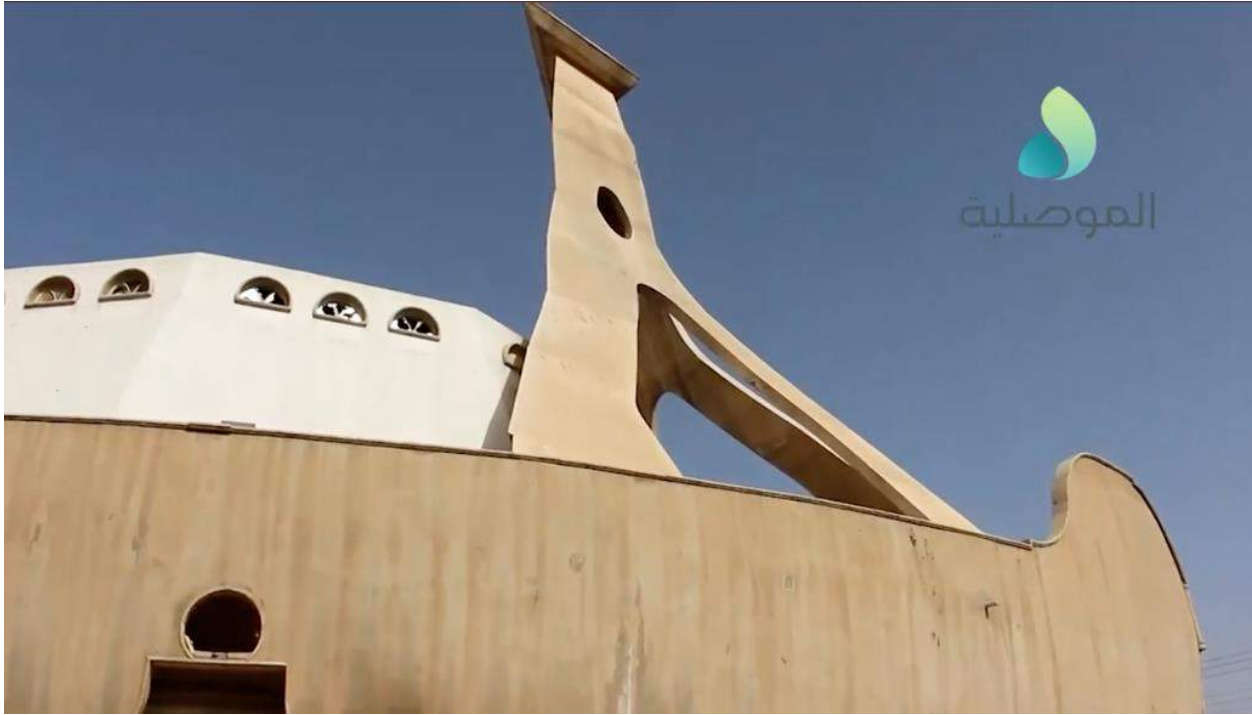
Video still of the exterior of the 'Ark Church' showing minimal damage, broken windows are seen (al-Mosuliya; January 11, 2017)
