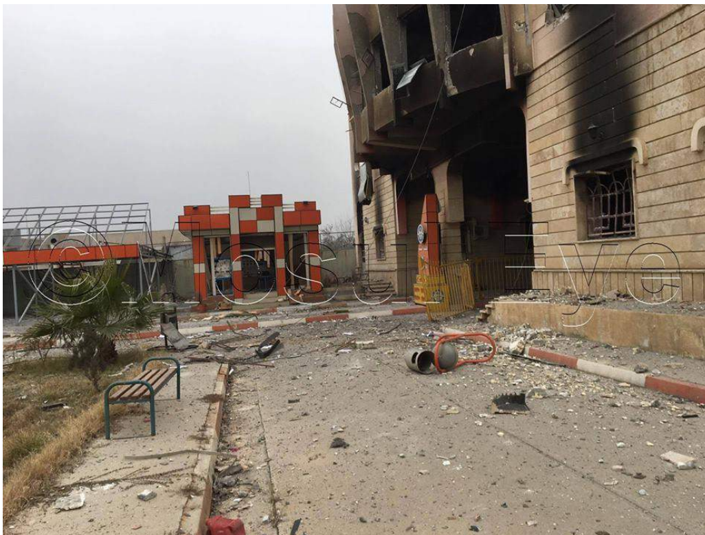
Detail of damage to the reported Technical College building at Mosul University (Mosul Eye; January 15, 2017)
