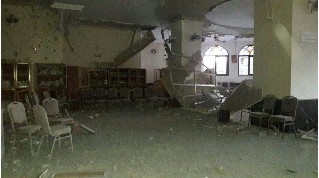
Damage to the building and furniture at the Northern Mosque in Madaya (SNHR; January 13, 2017)
