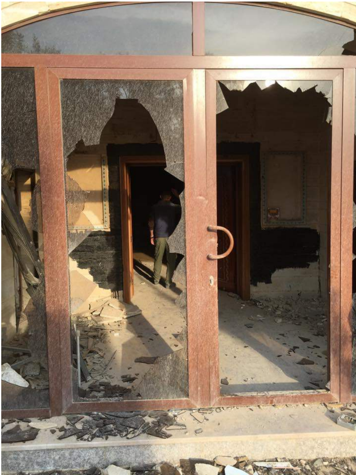
Damage to Mar Shmone Church (Twitter; January 22, 2017)
