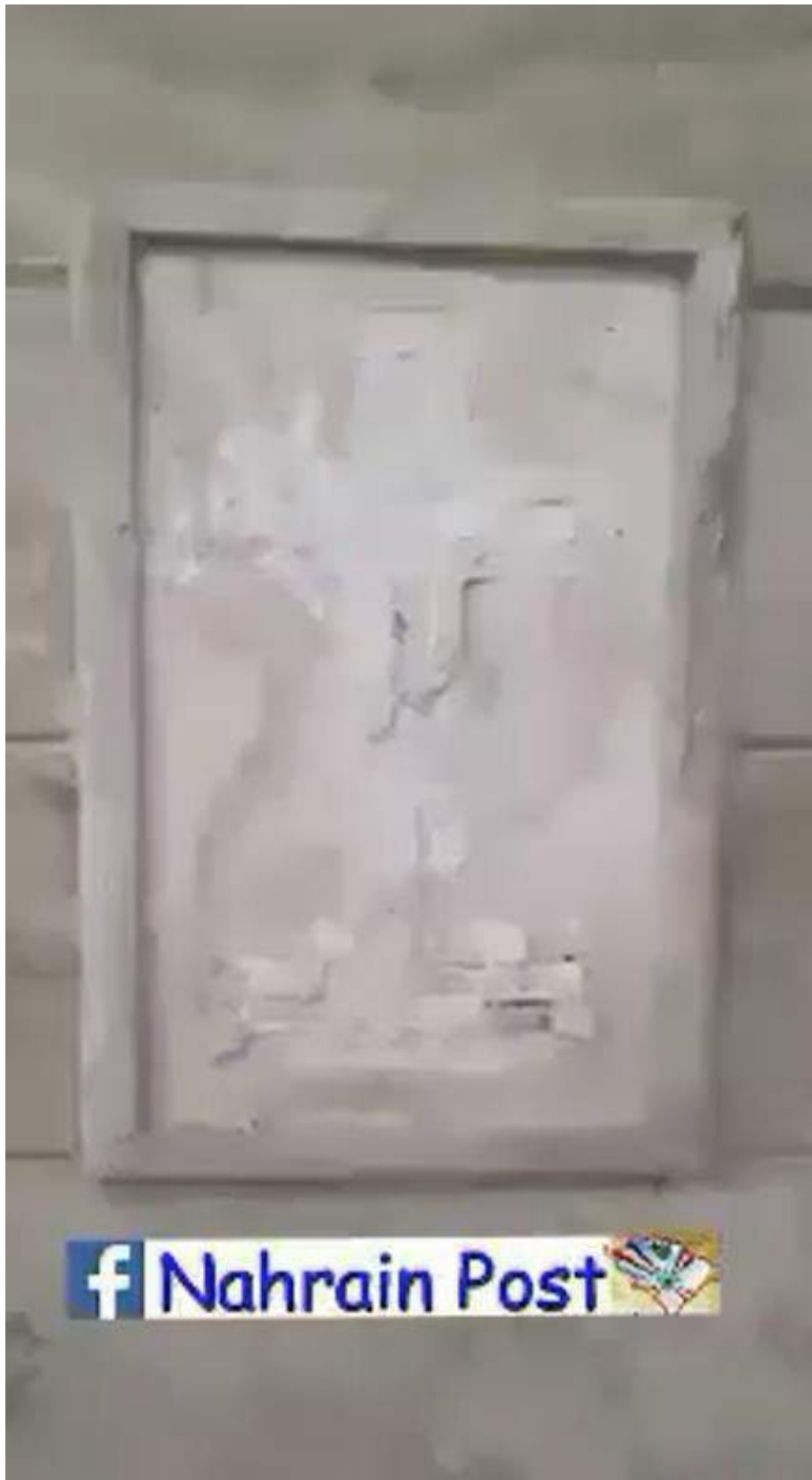
Damage to a cross on the exterior of Mar Yousif Church (Nahrain; January 24, 2017)
