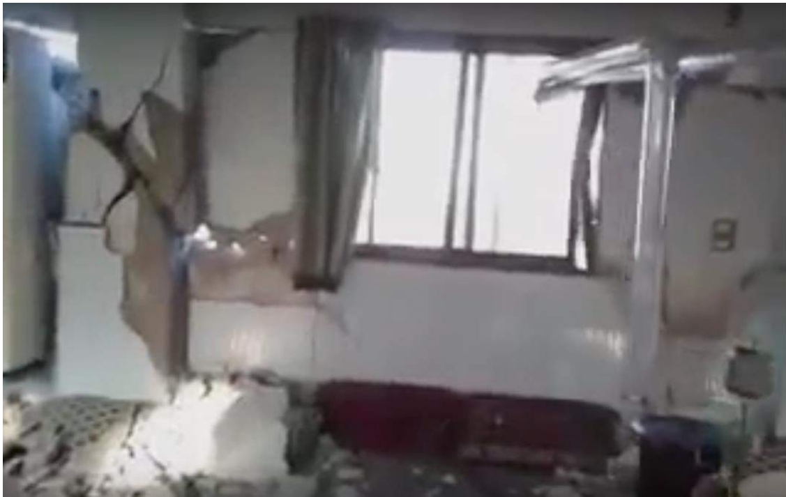
Video still of damage to interior of mosque (SNHR; January 30, 2017)
