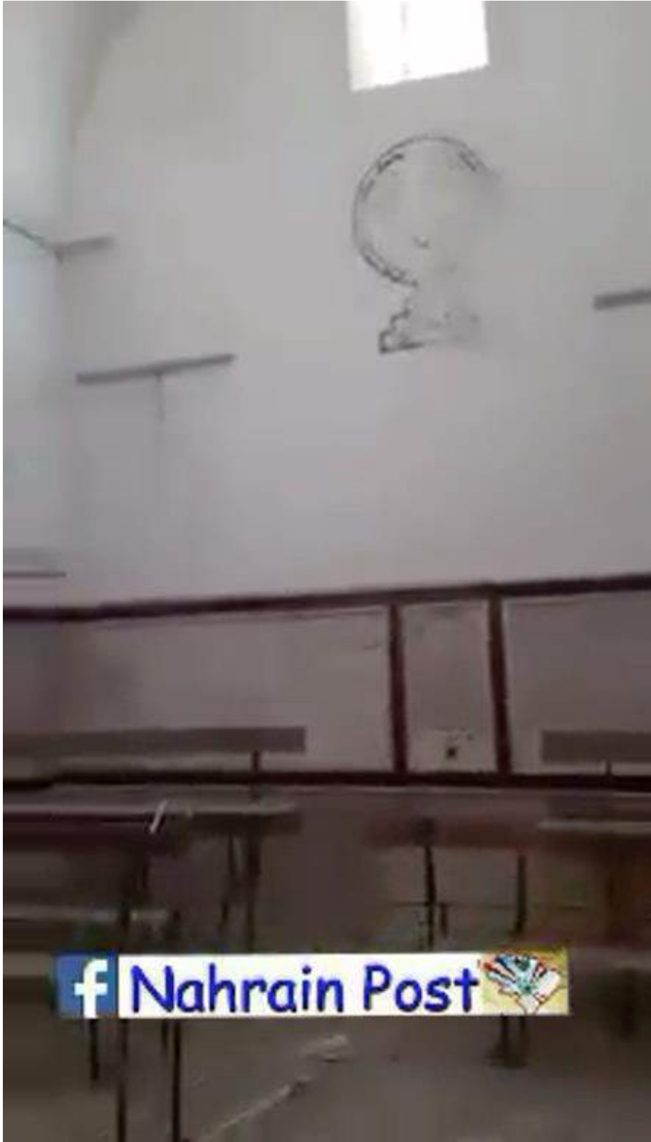
Damage to interior of Mar Yousif Church (Nahrain; January 24, 2017)
