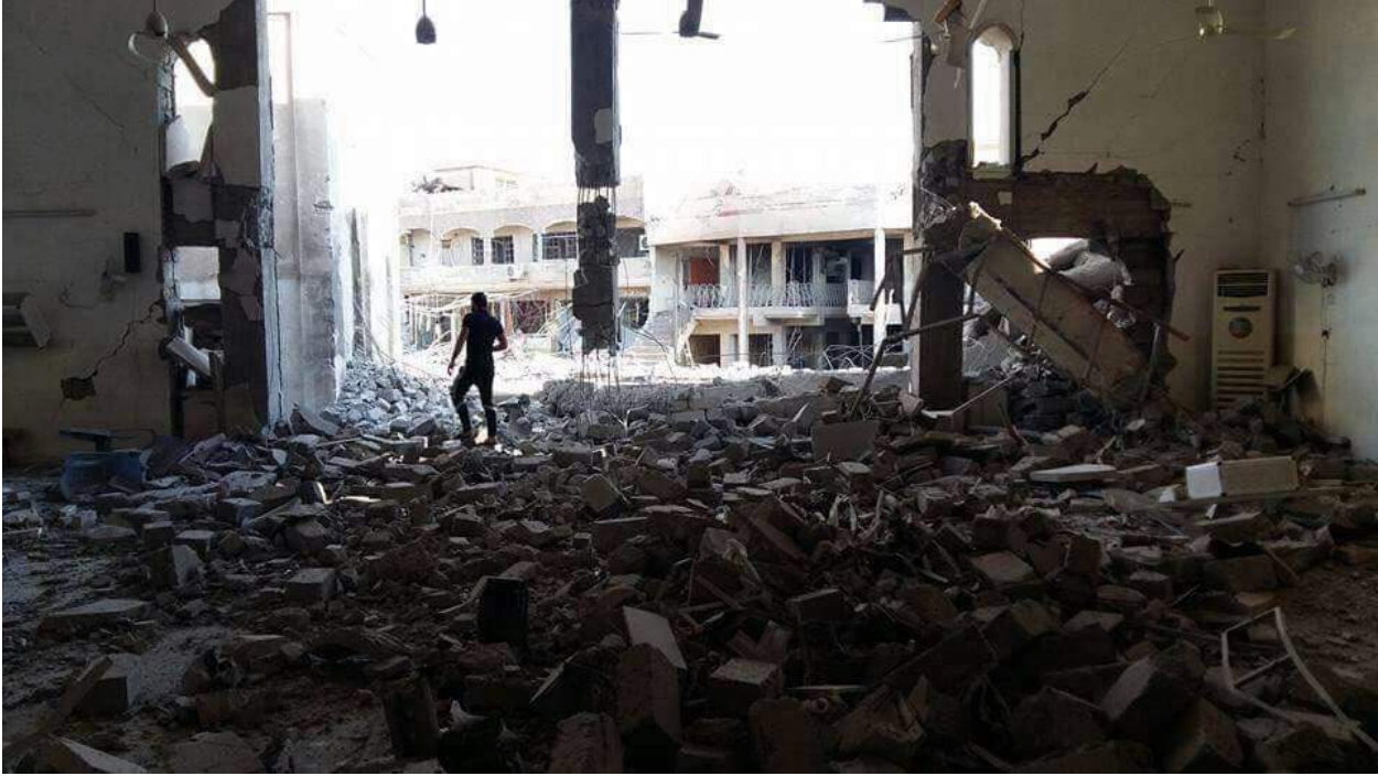
Missing front wall of al-Sayegh Mosque (DOAM; January 14, 2017)
