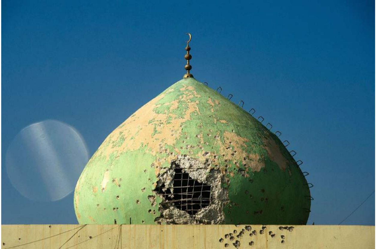
Damage to the dome of the al-Andalus Mosque (The Atlantic; January 19, 2017)
