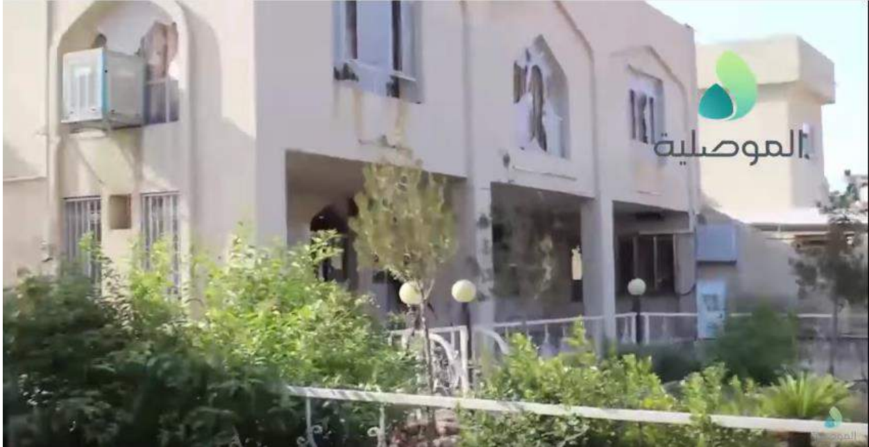
Video still of damage to the exterior of al-Rahman al-Rahim Mosque, broken windows visible (al-Mosuliya; January 11, 2017)
