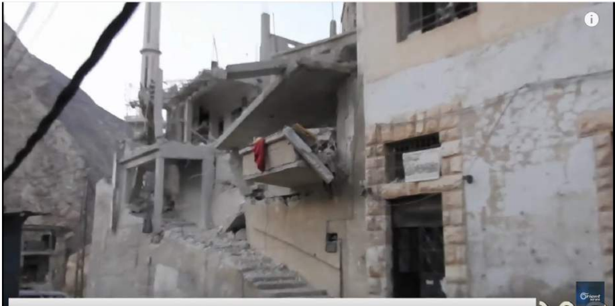
Damage to Ein al-Khadra Mosque and surrounding buildings (Orient News; January 7, 2016)
