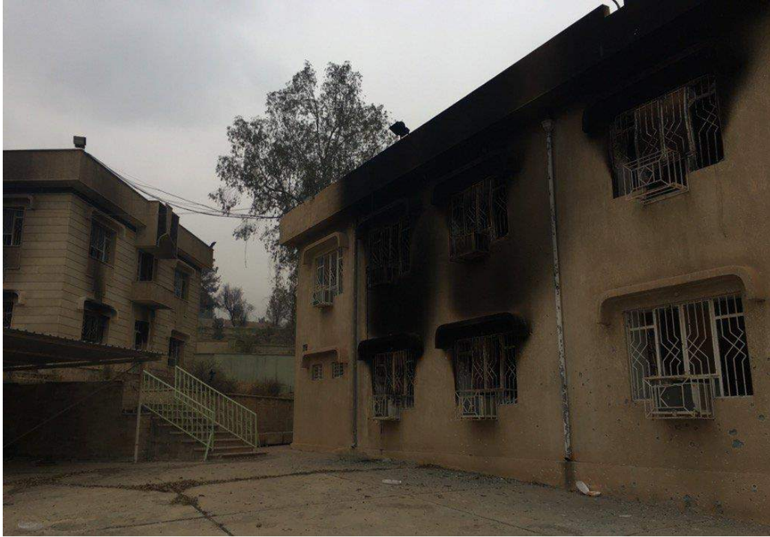
A burned out building at Mosul University (W.G. Dunlop; January 20, 2017)
