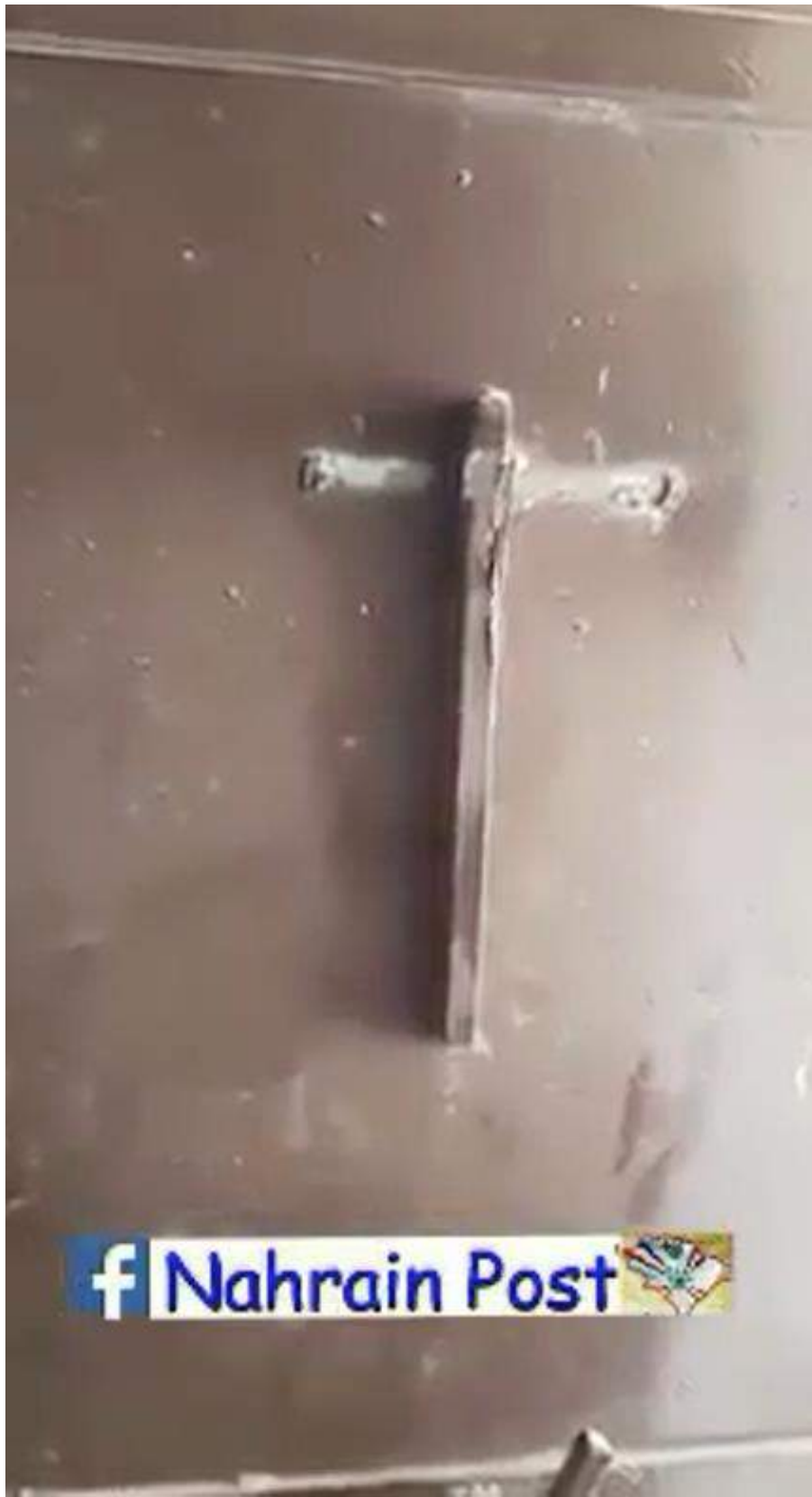
Damage to a cross at Mar Yousif Church (Nahrain; January 24, 2017)
