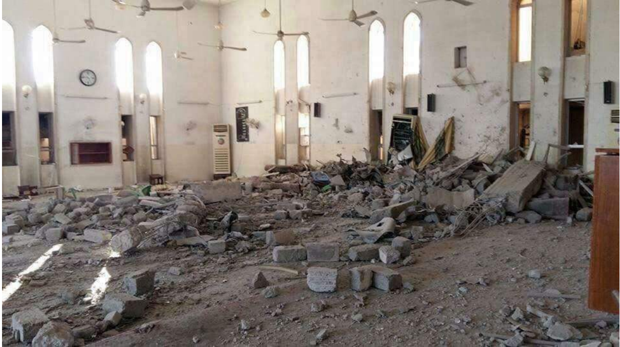
Rubble inside the al-Sayegh Mosque (DOAM; January 14, 2017)
