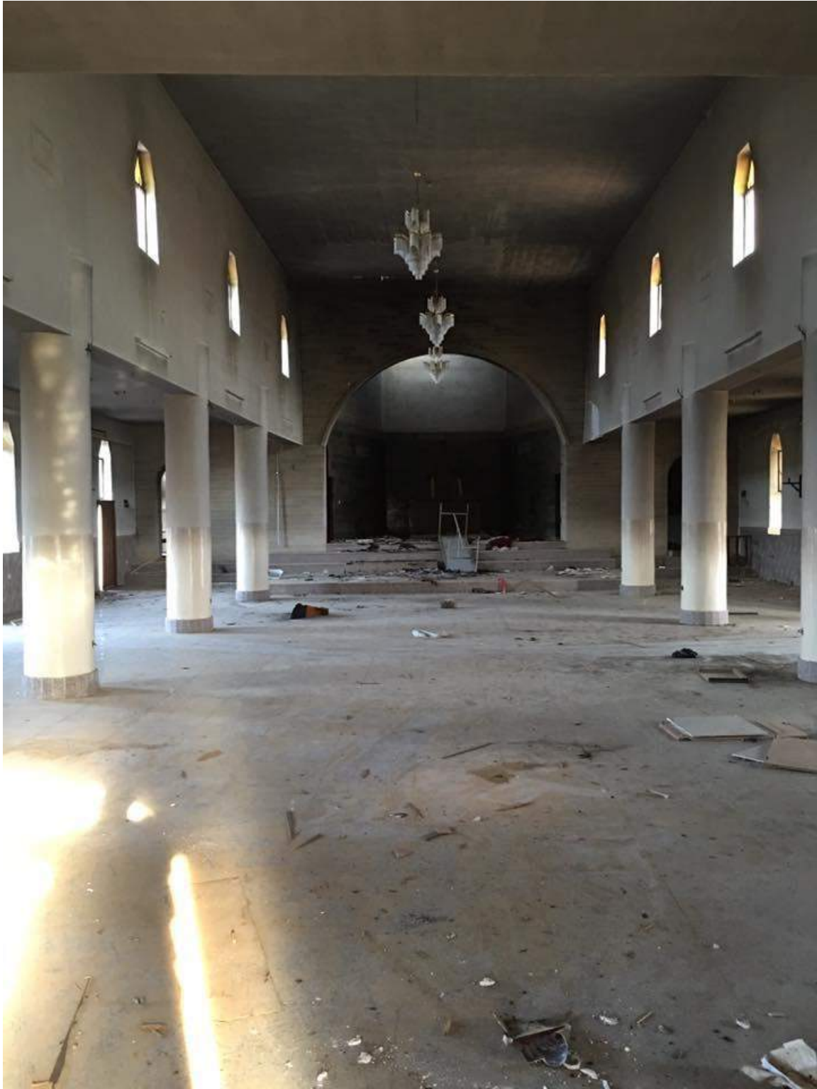
Damage inside Mar Shmone Church (Twitter; January 22, 2017)
