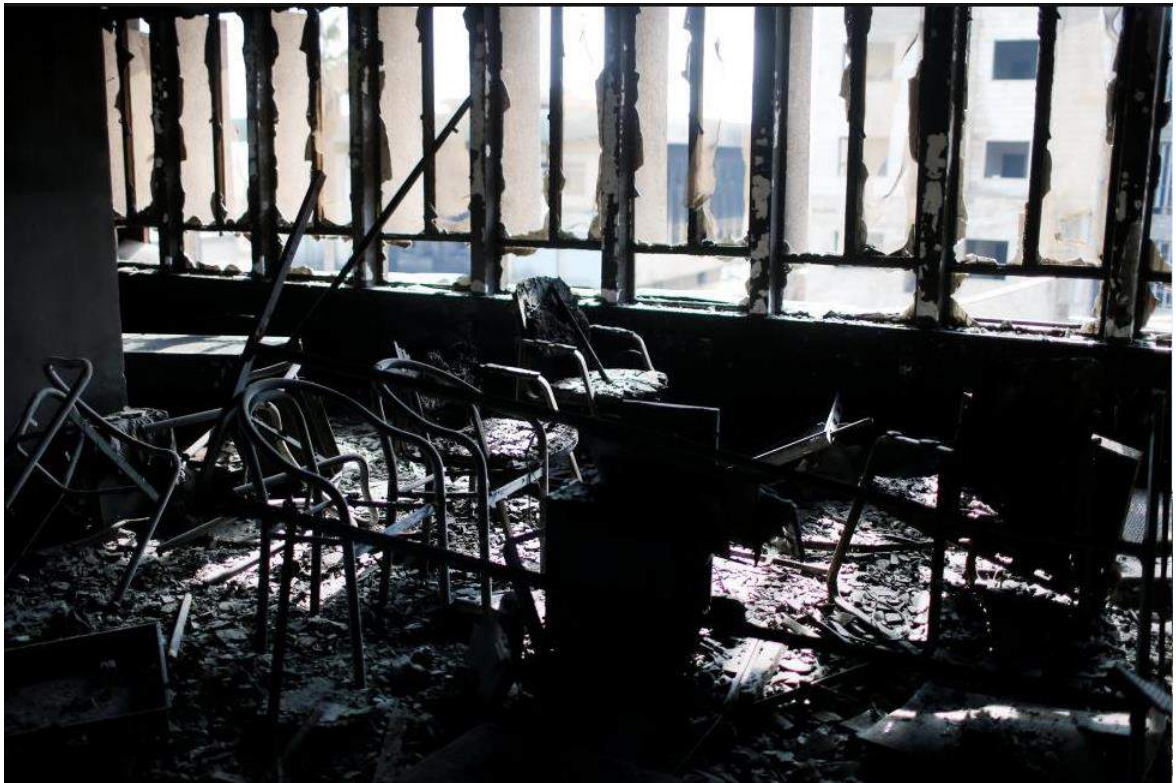
Damage seen at the Central Library (Reuters; January 31, 2017)
