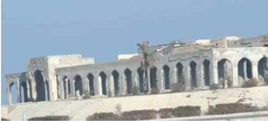
Damage seen to the exterior of the Nebi Yunus Mosque Complex (Iraqi News; January 26, 2017)
