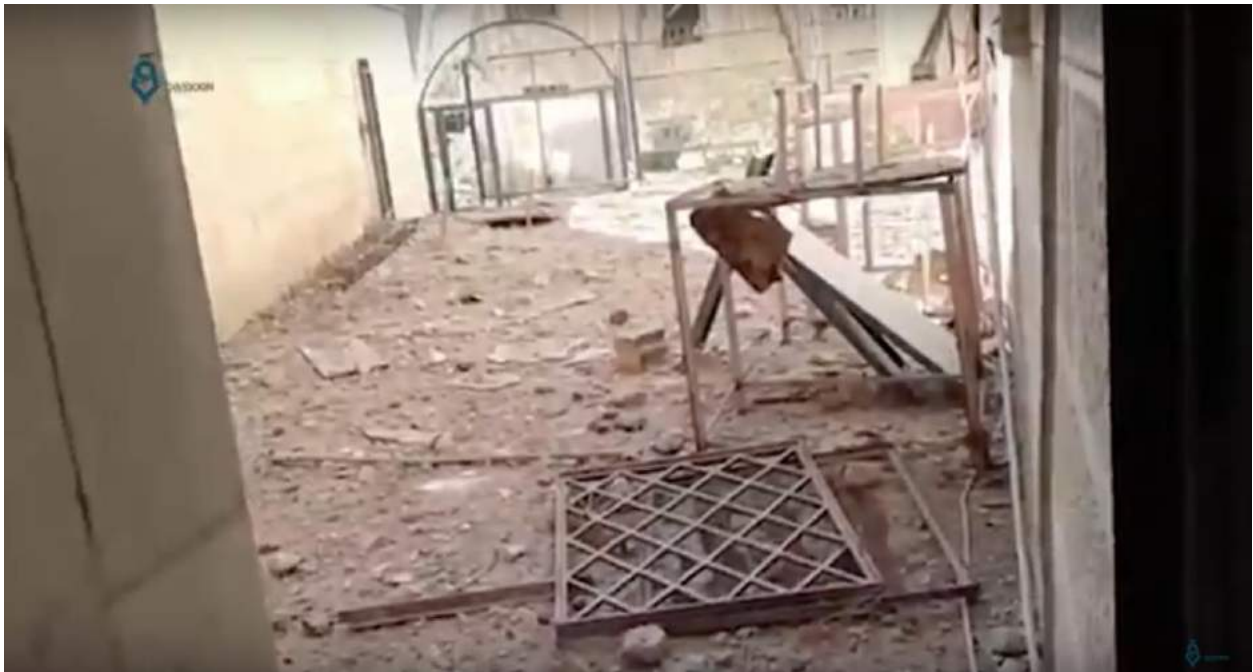
Video still of damage to courtyard of al-Mahmoudi Mosque (Qasioun News; January 25, 2017)
