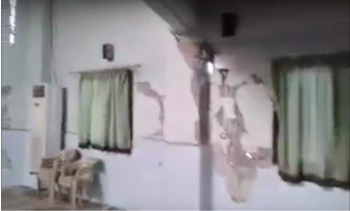
Video still of damage to interior of mosque (SNHR; January 30, 2017)
