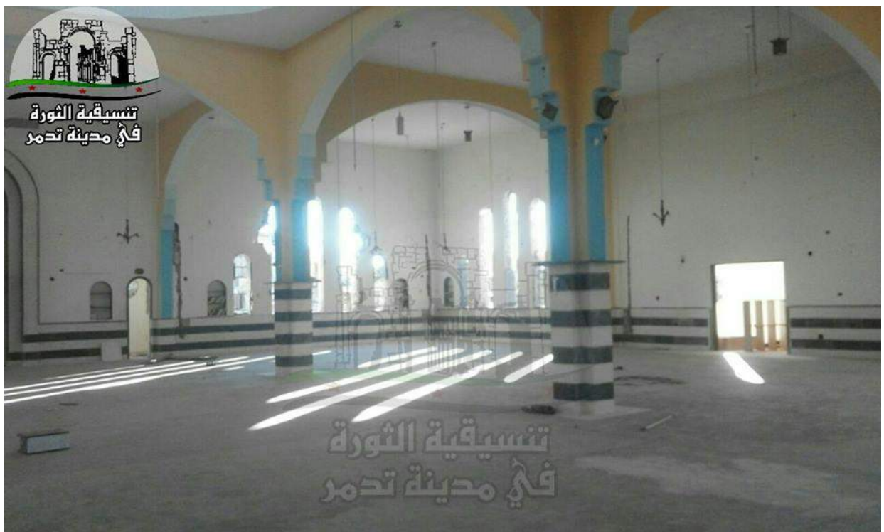
Damage to the interior of Abi Thar al-Ghafari Mosque (Palmyra Coordination Committee; January 9, 2017)
