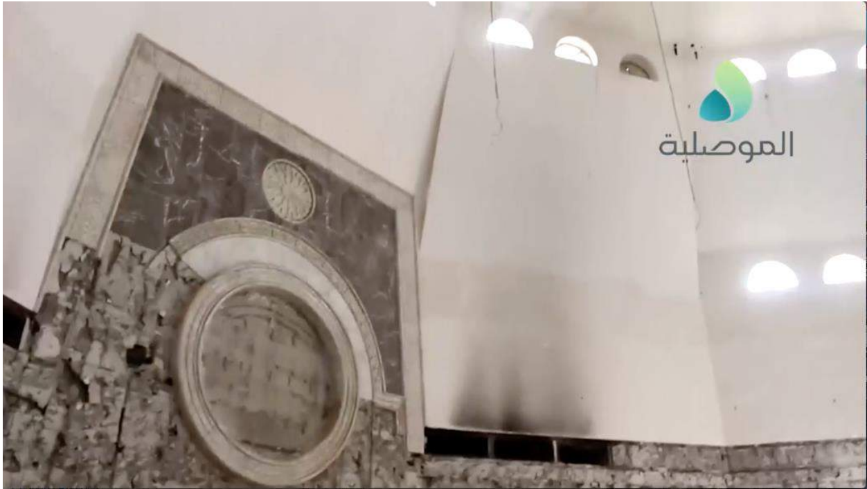
Video still of damage to the interior of the church (al-Mosuliya; January 11, 2017)
