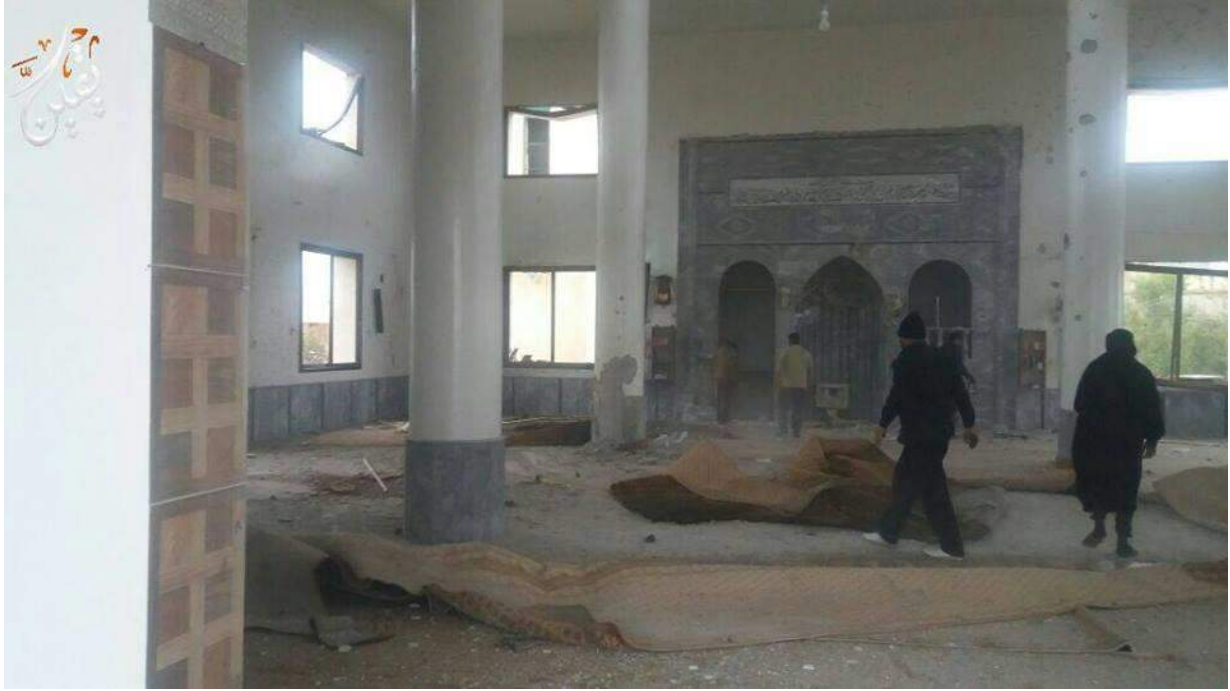
Damage to the interior of al-Khalaf Mosque (SNHR; January 14, 2017)
