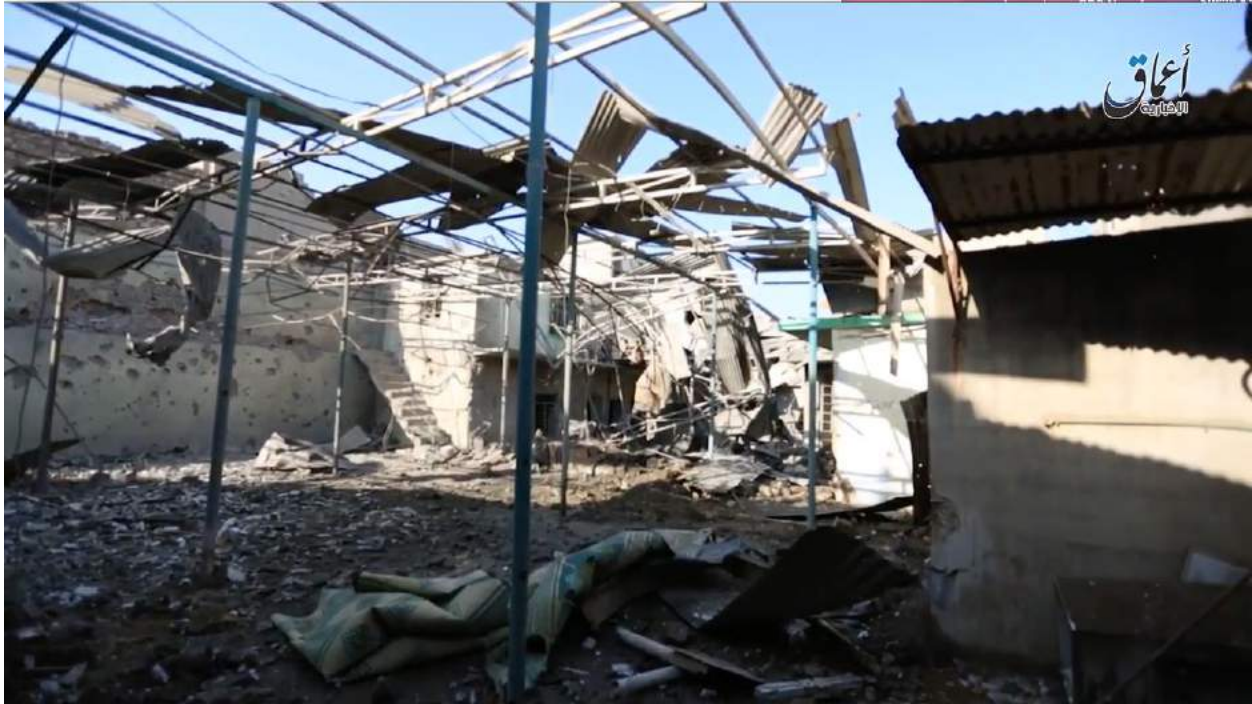
Video still of extensive damage to the exterior of al-Khatib Mosque (Amaq News Agency; December 23, 2016)
