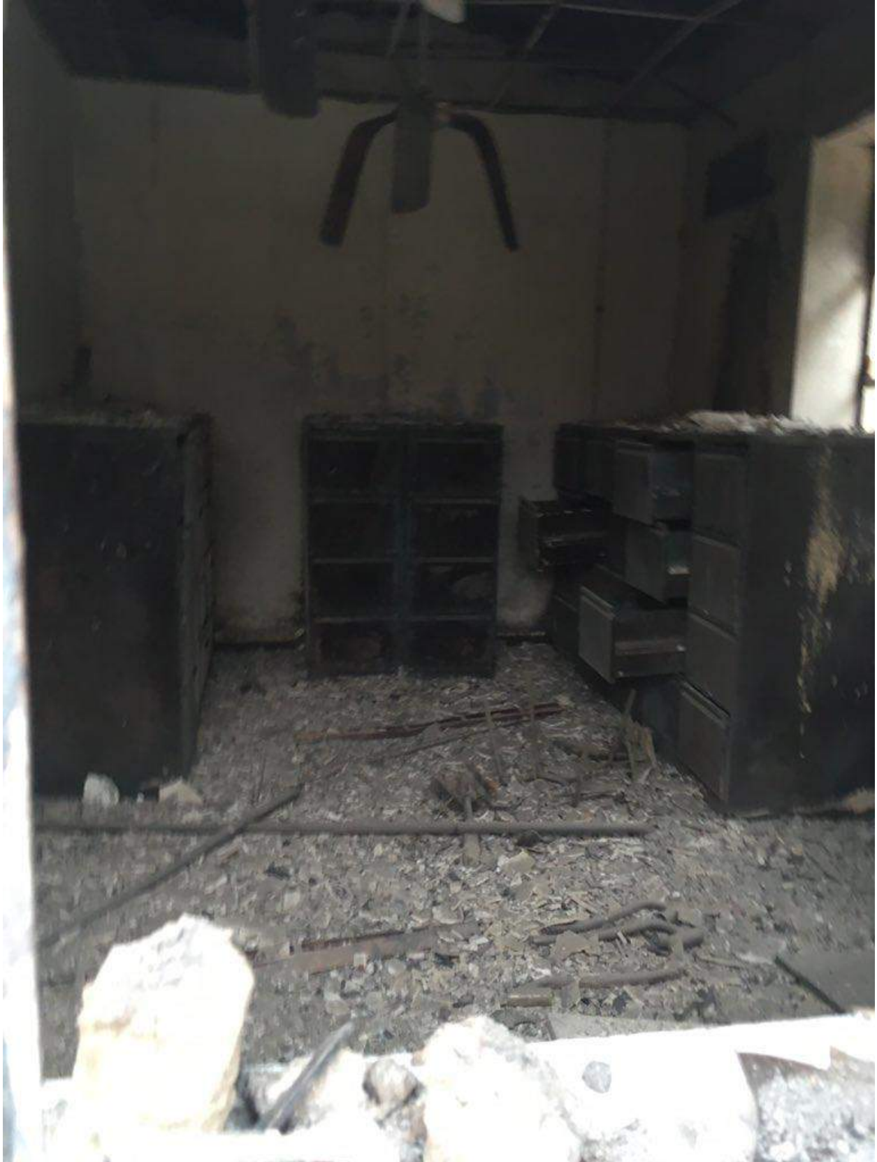
Damage seen inside a Mosul University building (W.G. Dunlop; January 16, 2017)
