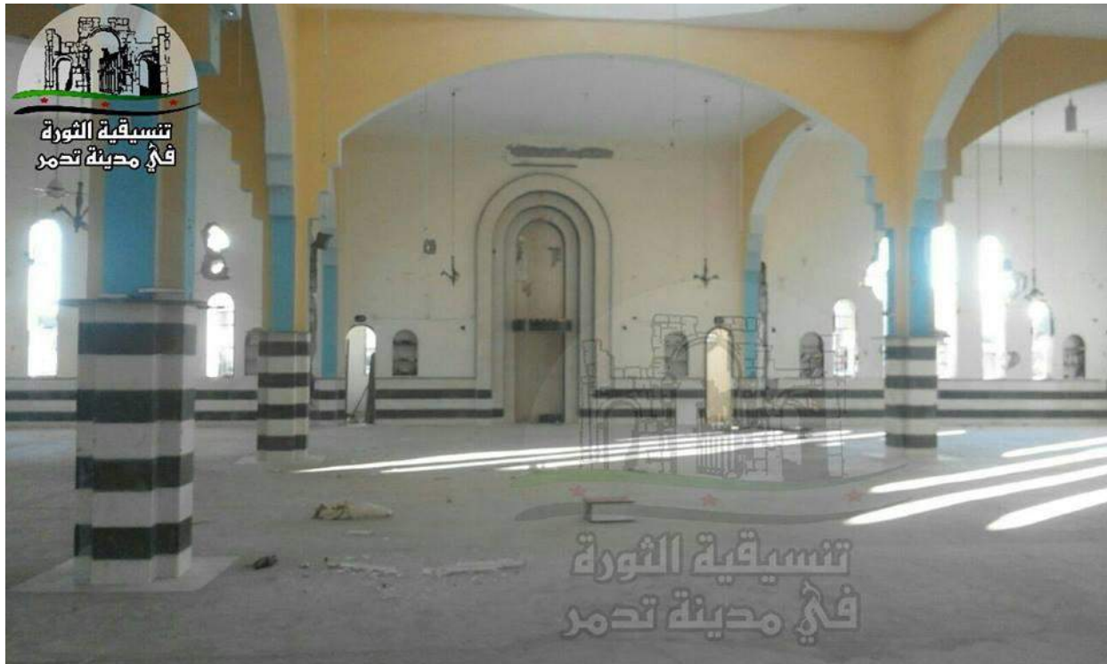
Damage to the interior of Abi Thar al-Ghafari Mosque (Palmyra Coordination Committee; January 9, 2017)
