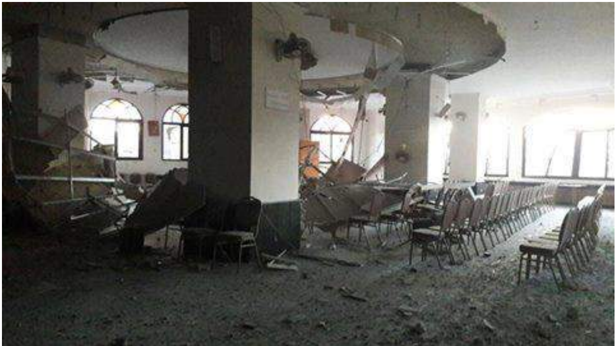
Damage to the Northern Mosque in Madaya (Syrian Revolution Network; January 12, 2017)
