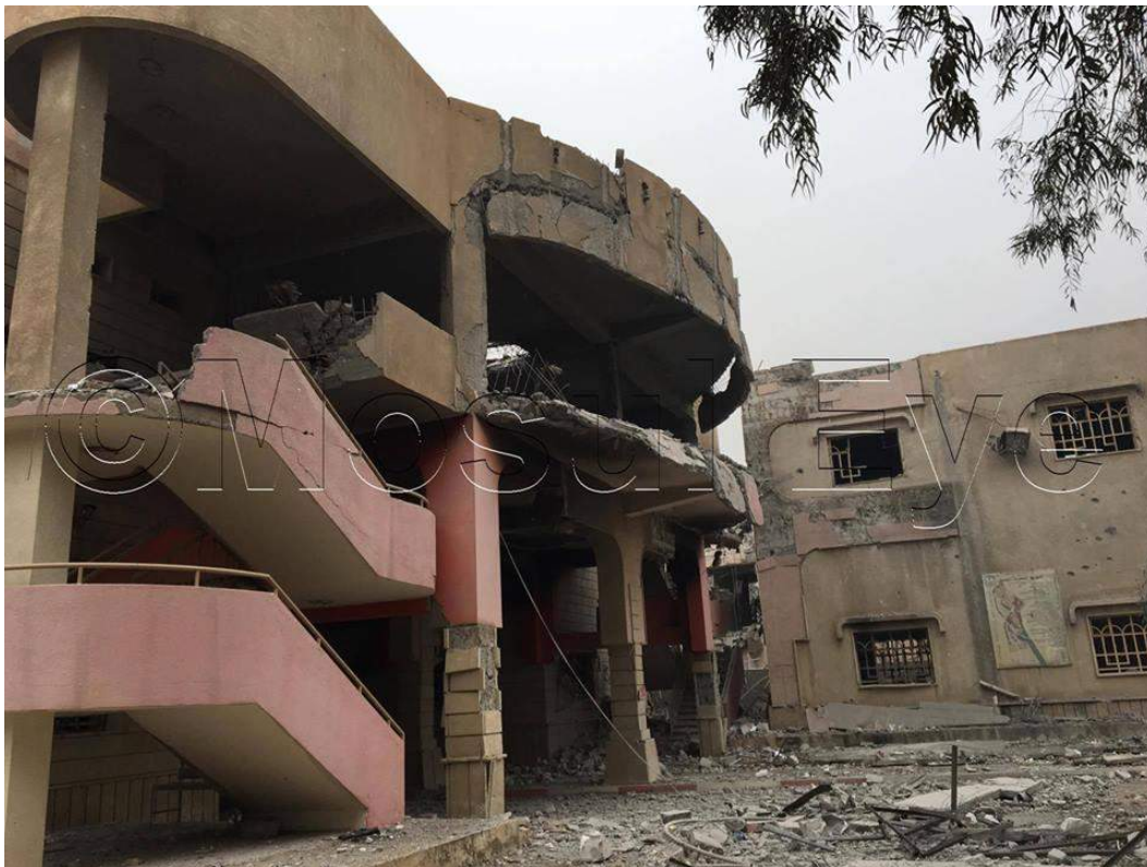
Damage to a campus building at Mosul University (Mosul Eye; January 15, 2017)
