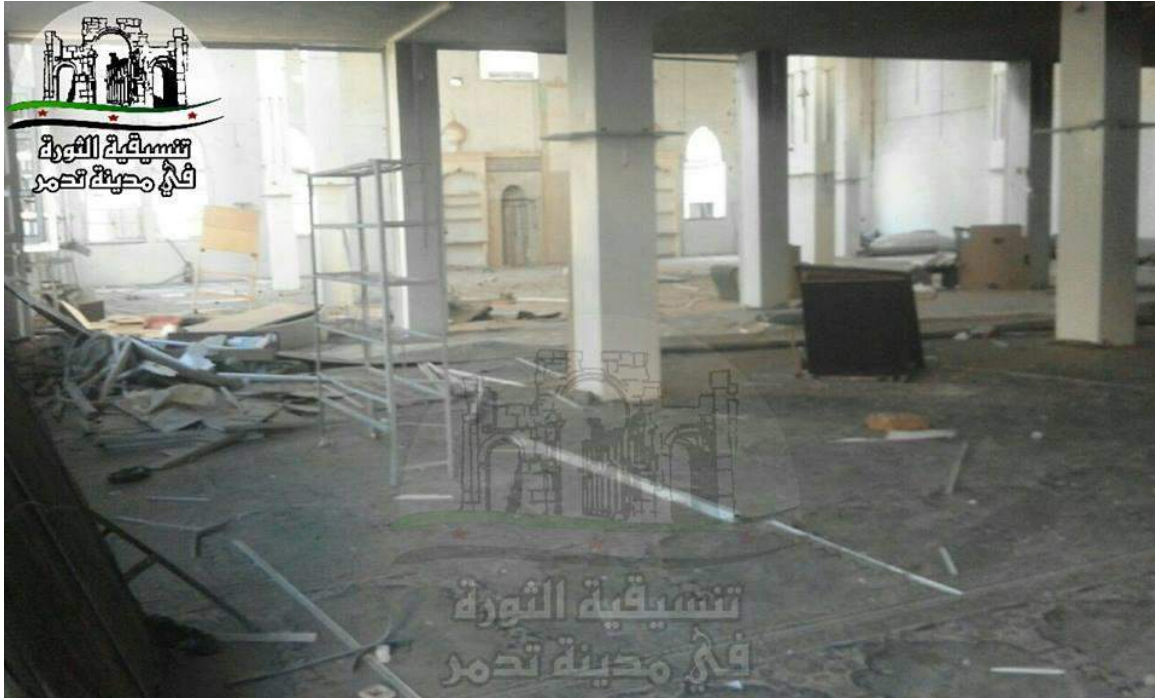
Damage to the inside of al-Eman Mosque in Palmyra (Palmyra Coordination; January 6, 2017)
