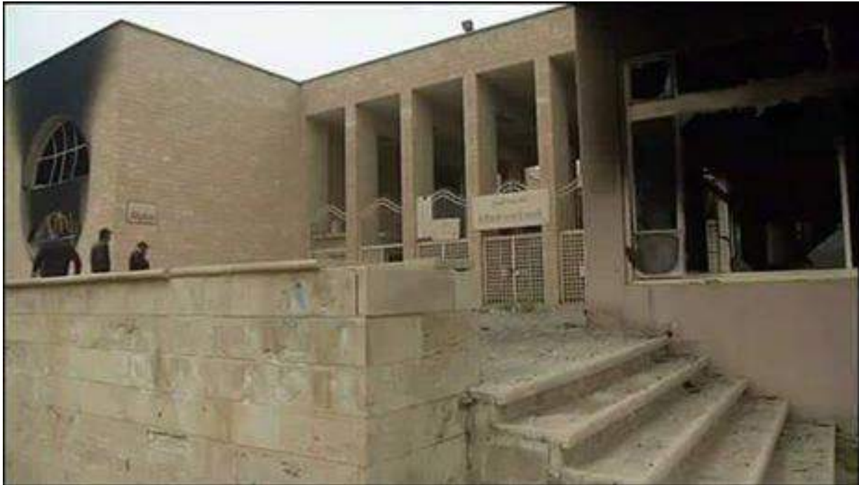
Fire damage seen at Mosul University Student Center (مجتهد الأنبار; January 16, 2016)
