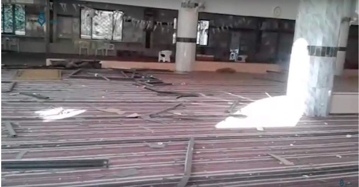
Video still of damage to interior of al-Mahmoudi Mosque (Qasioun News; January 25, 2017)
