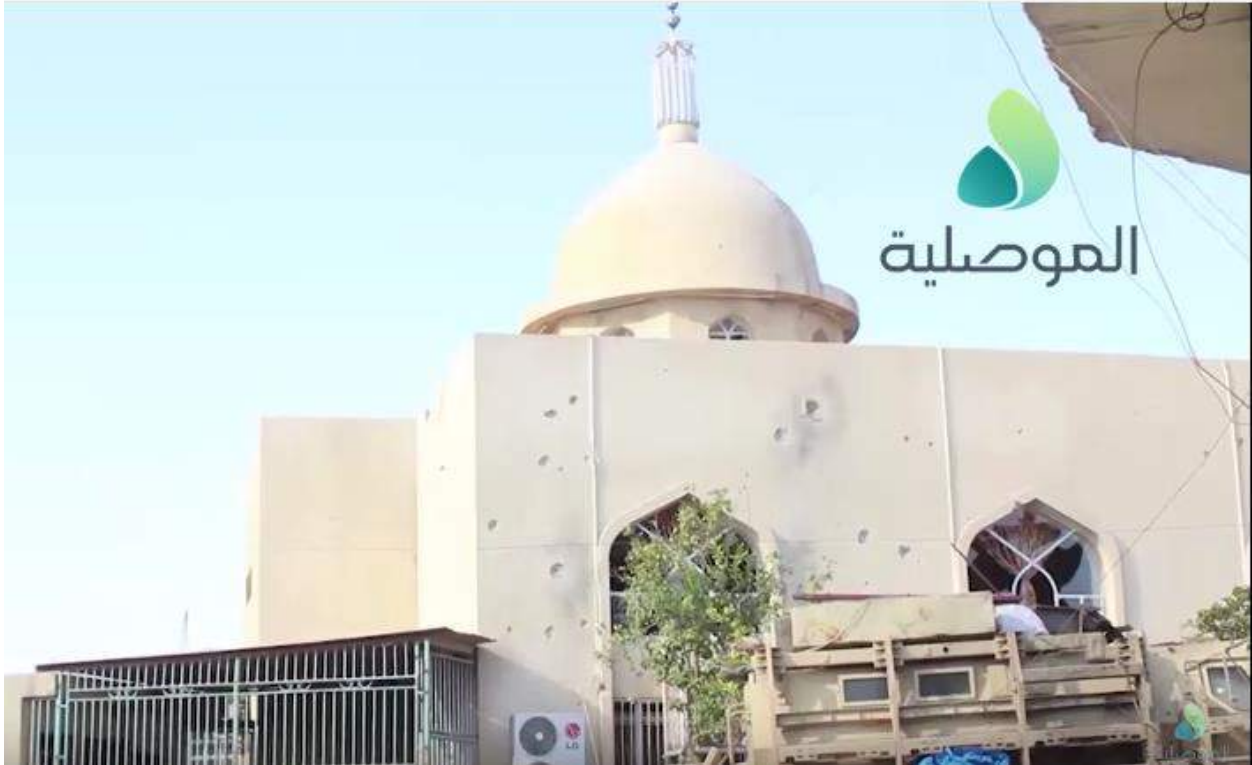
Video still showing damage to the exterior of al-Rahman al-Rahim Mosque (al-Mosuliya; January 11, 2017)
