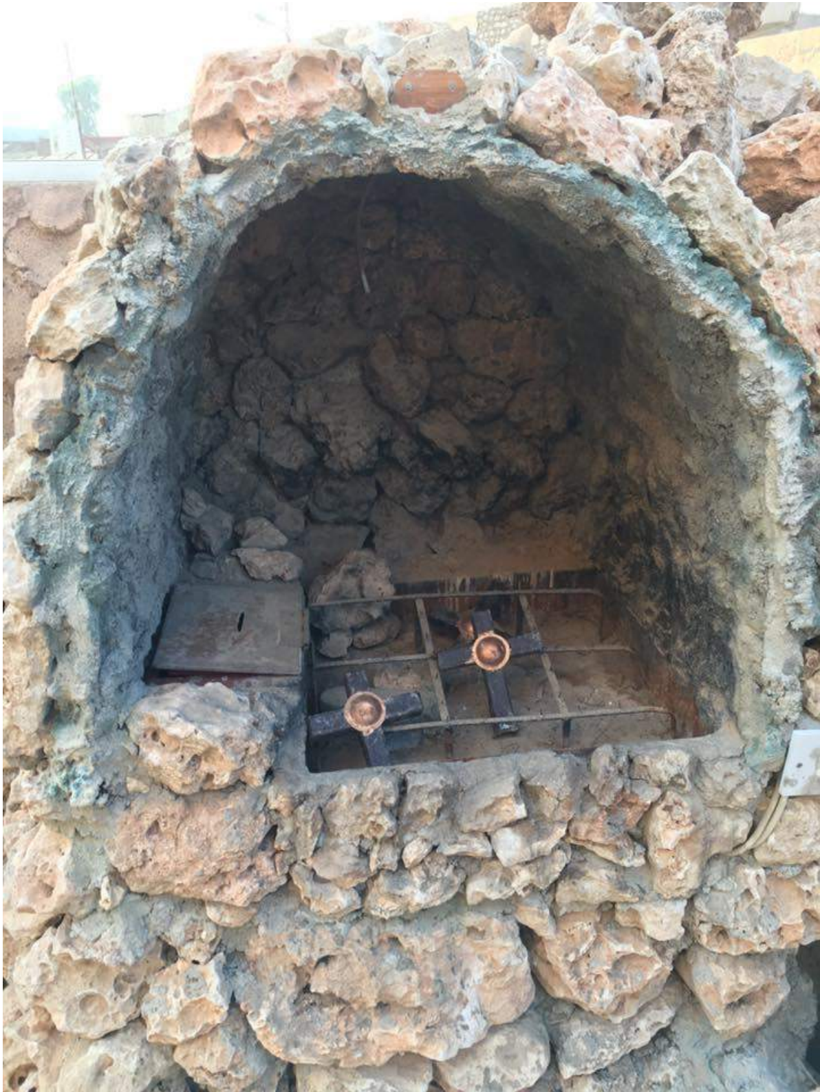
Damage seen to Mar Shmone Church (Twitter; January 22, 2017)
