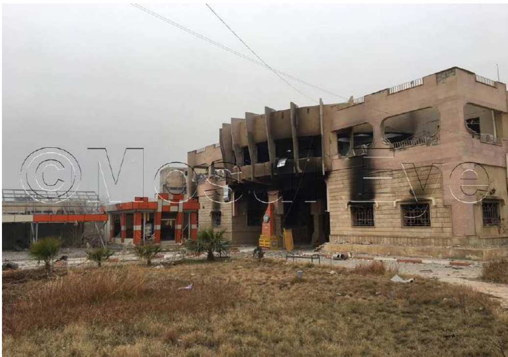
Damage to the reported Technical College building at Mosul University (Mosul Eye; January 15, 2017)
