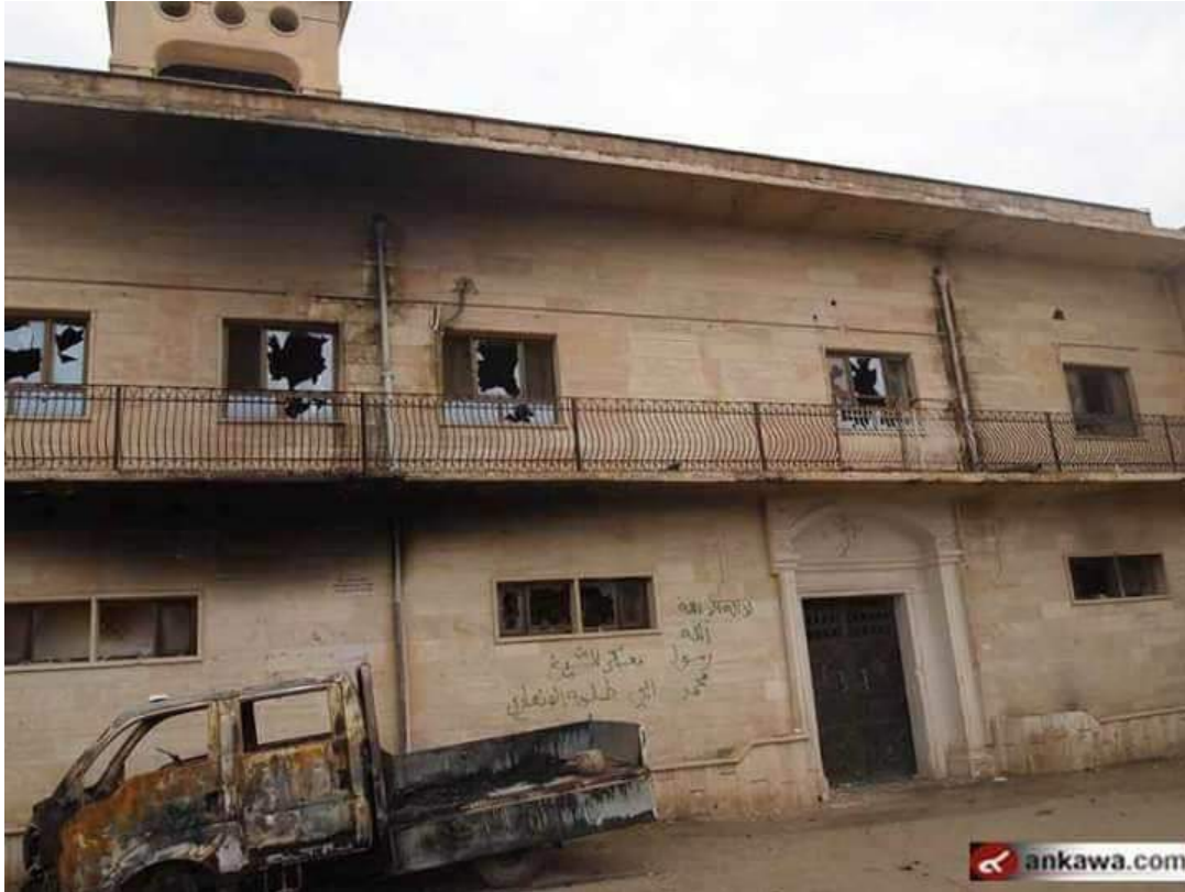
Damage, including broken glass and graffiti, seen at Sacred Heart Church (Nahrain; January 24, 2017)
