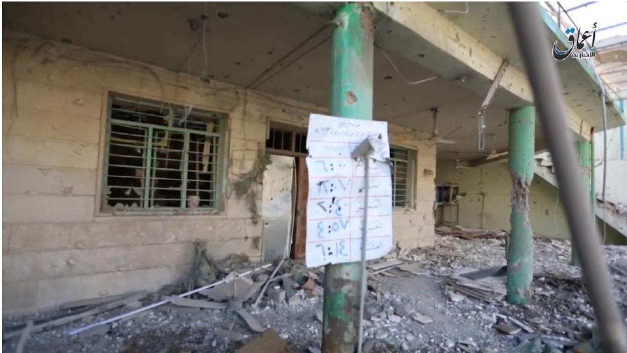
Video still of extensive damage to the exterior of al-Khatib Mosque, prayer times exhibited in the center of the still (Amaq News Agency; December 23, 2016)
