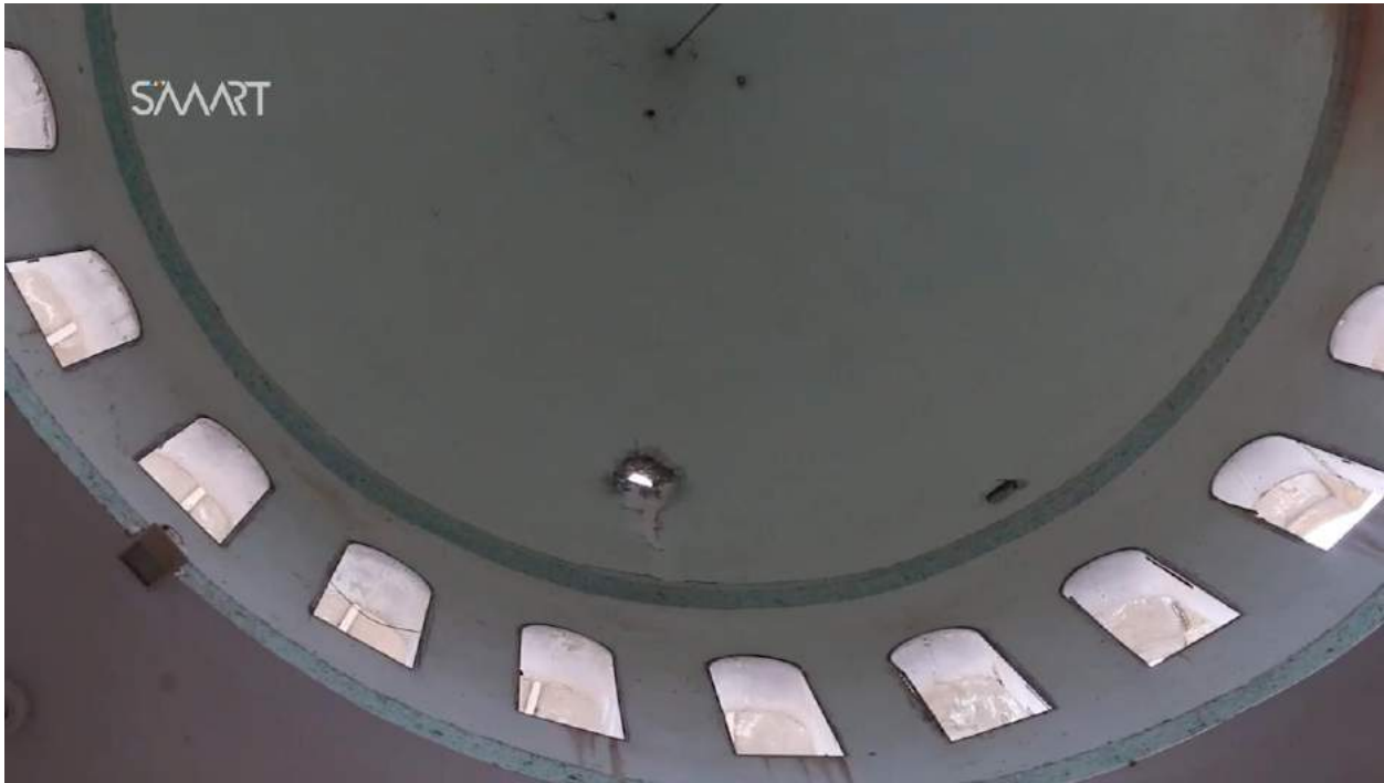
Video still of damage to the dome of Usama bin Zaid Mosque (Smart News Agency; April 14, 2017)
