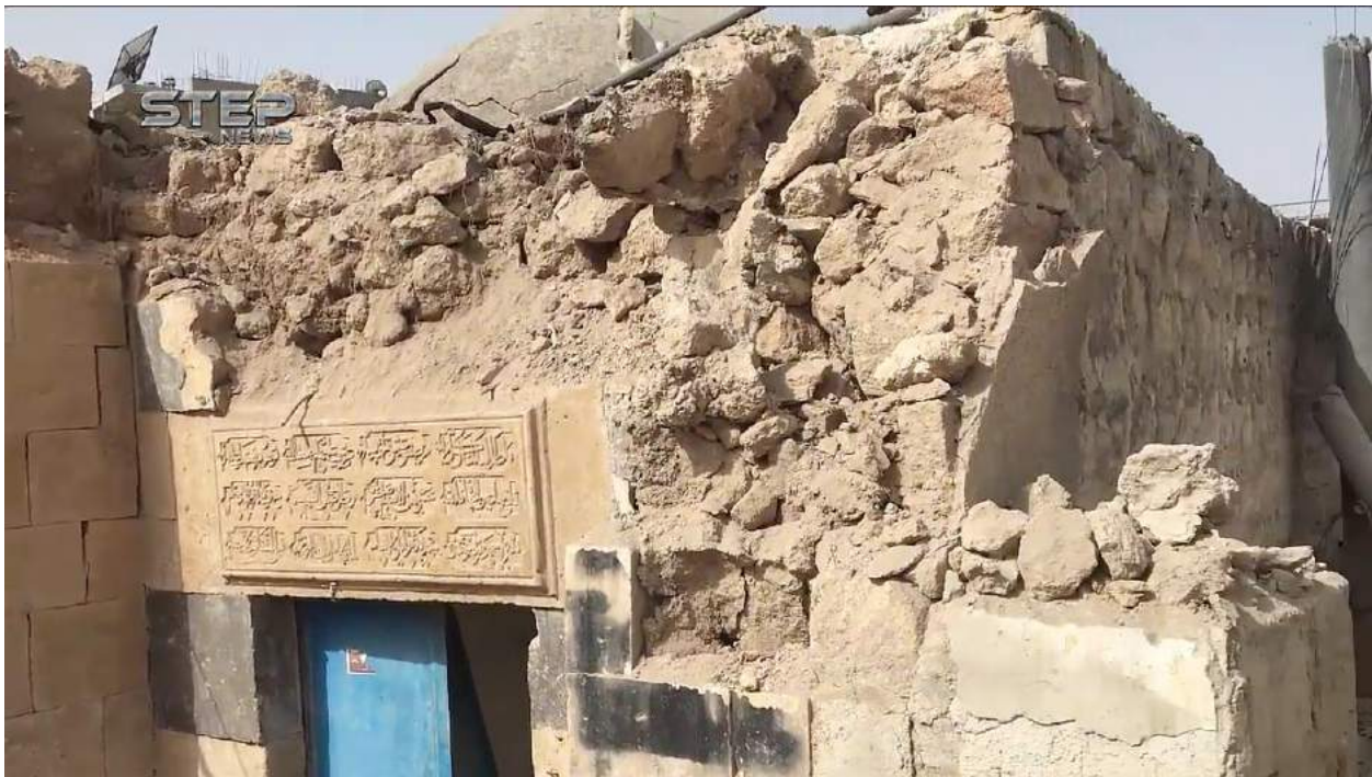
Video still of severe damage to Hammam al-Daraj al-Qadim (Step News Agency; April 27, 2017)
