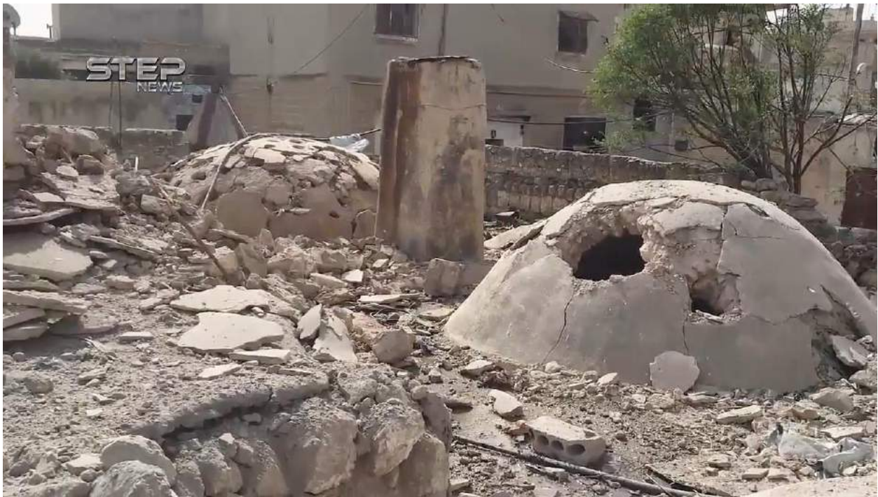
Video still of severe damage to Hammam al-Daraj al-Qadim (Step News Agency; April 27, 2017)
