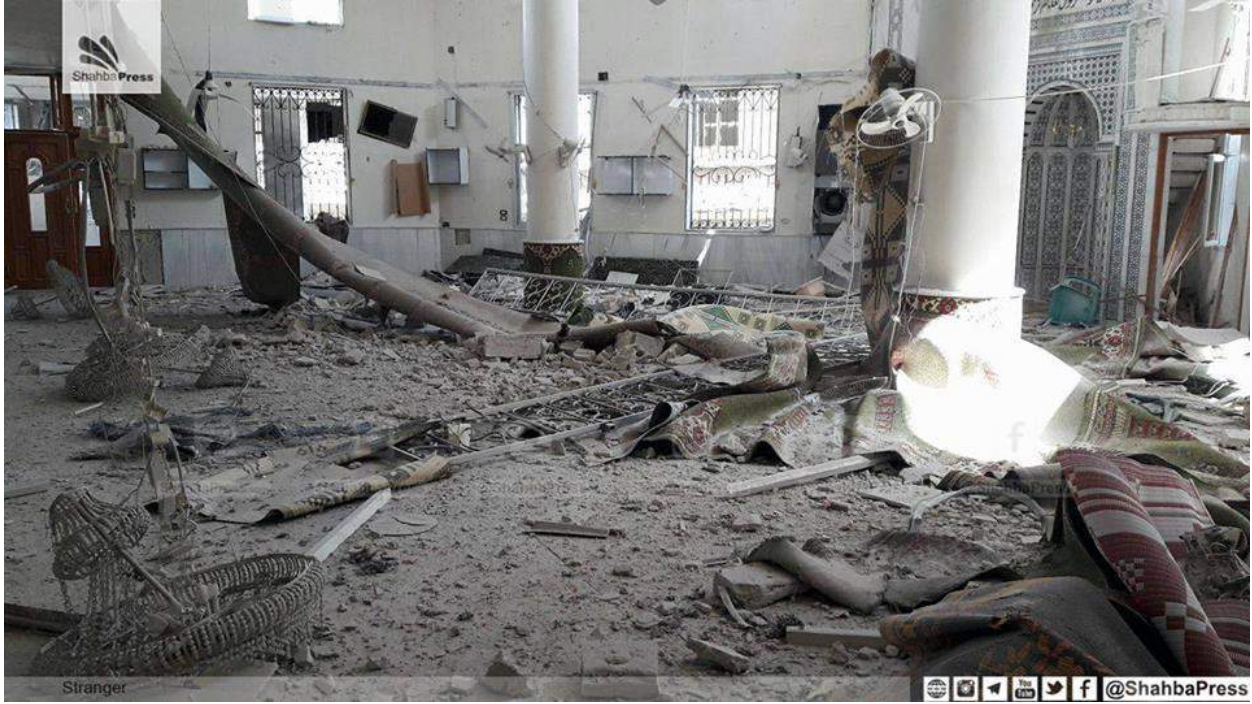
Damage to interior of al-Sahabat al-Abrar Mosque (Shahba Press Agency; April 10, 2017)
