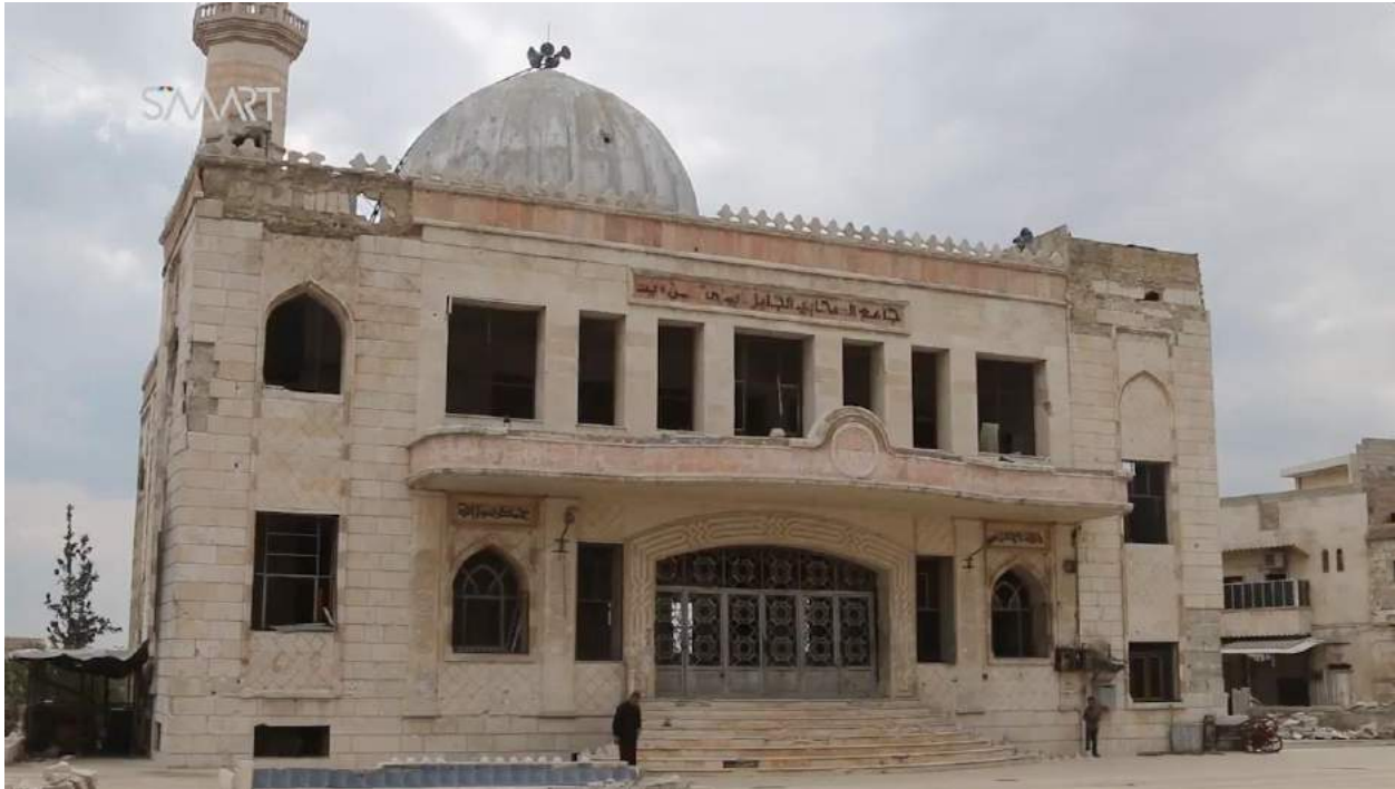
Video still of damage to the exterior of Usama Bin Zaid Mosque (Smart News Agency; April 14, 2017)
