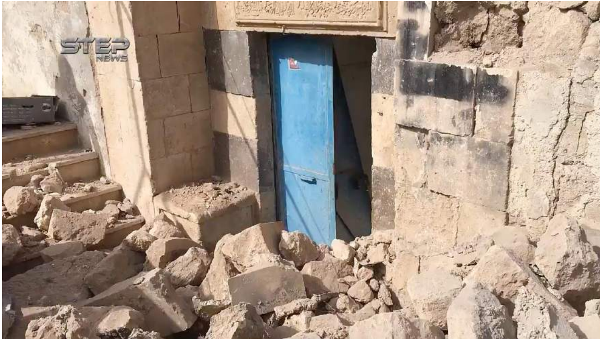
Video still of severe damage to Hammam al-Daraj al-Qadim (Step News Agency; April 27, 2017)
