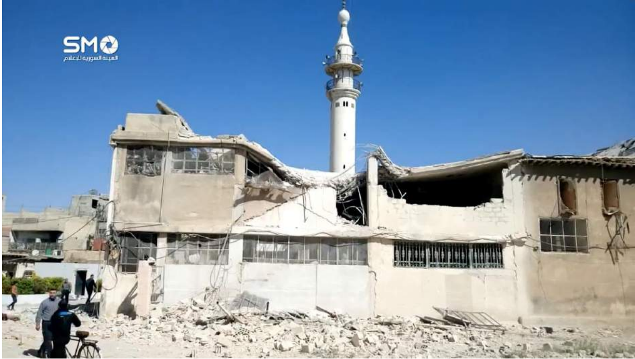
Video still of extensive damage to Arbin al-Kabir Mosque (SMO Syria; April 8, 2017)
