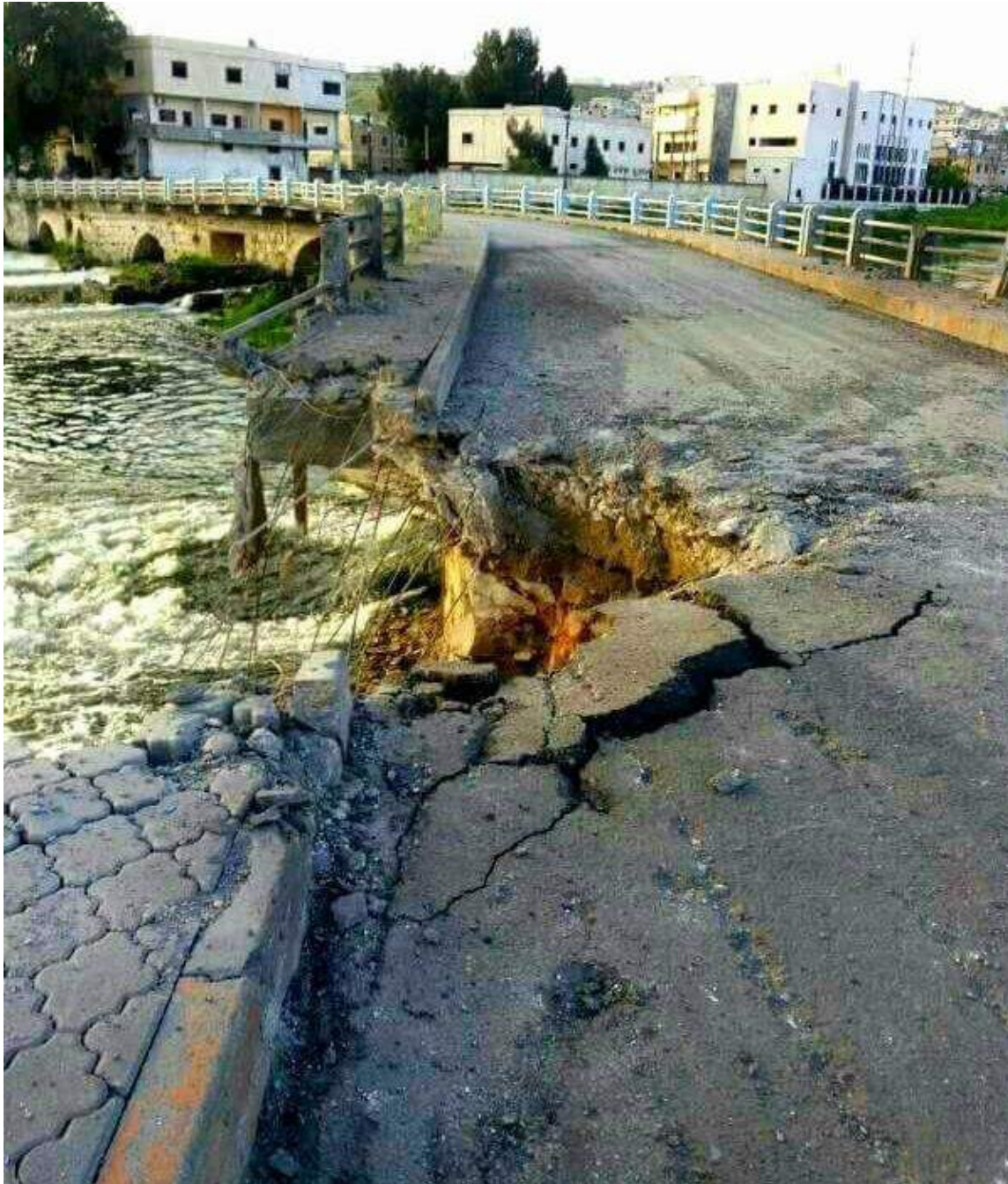
Damage to the Roman bridge (Idlib Antiquities Center; April 8, 2017)
