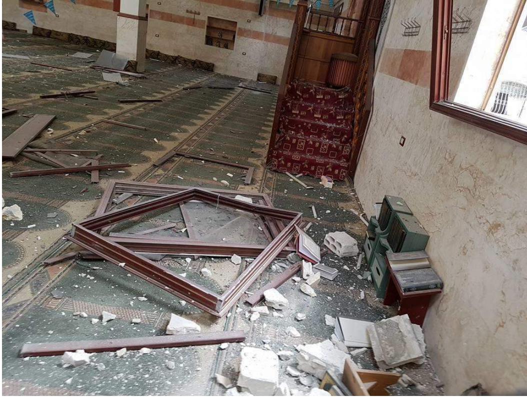
Damage to the interior of Hamza Bin Abd al-Mutalleb Mosque (SNHR; April 8, 2017)
