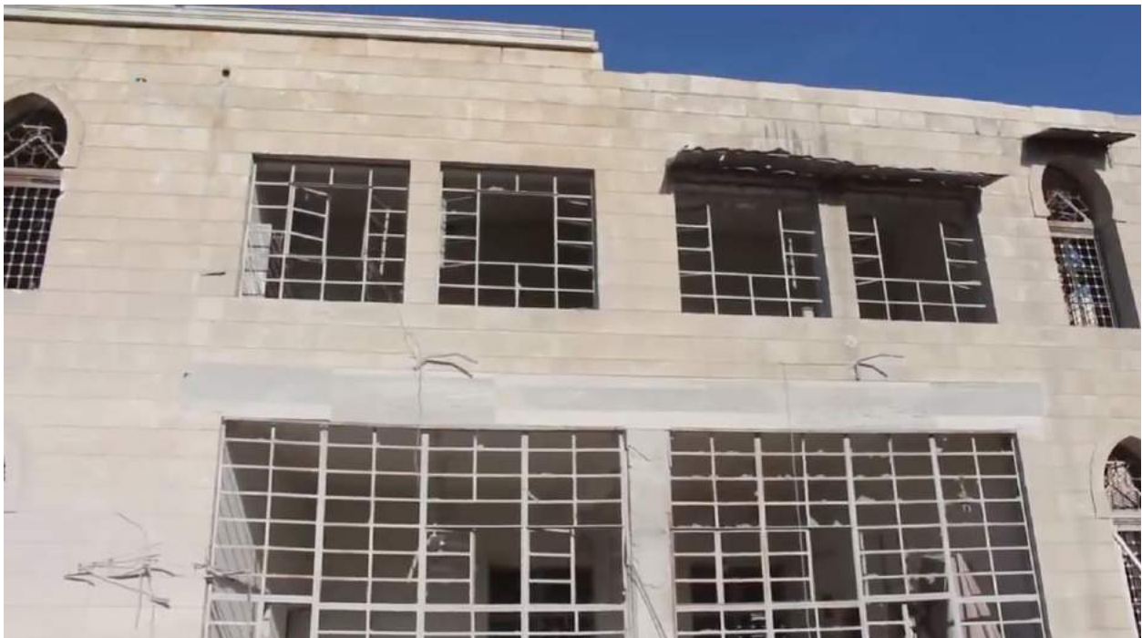
Video still shows damage to al-Rawda Mosque (Salqin City Coordination; April 7, 2017)
