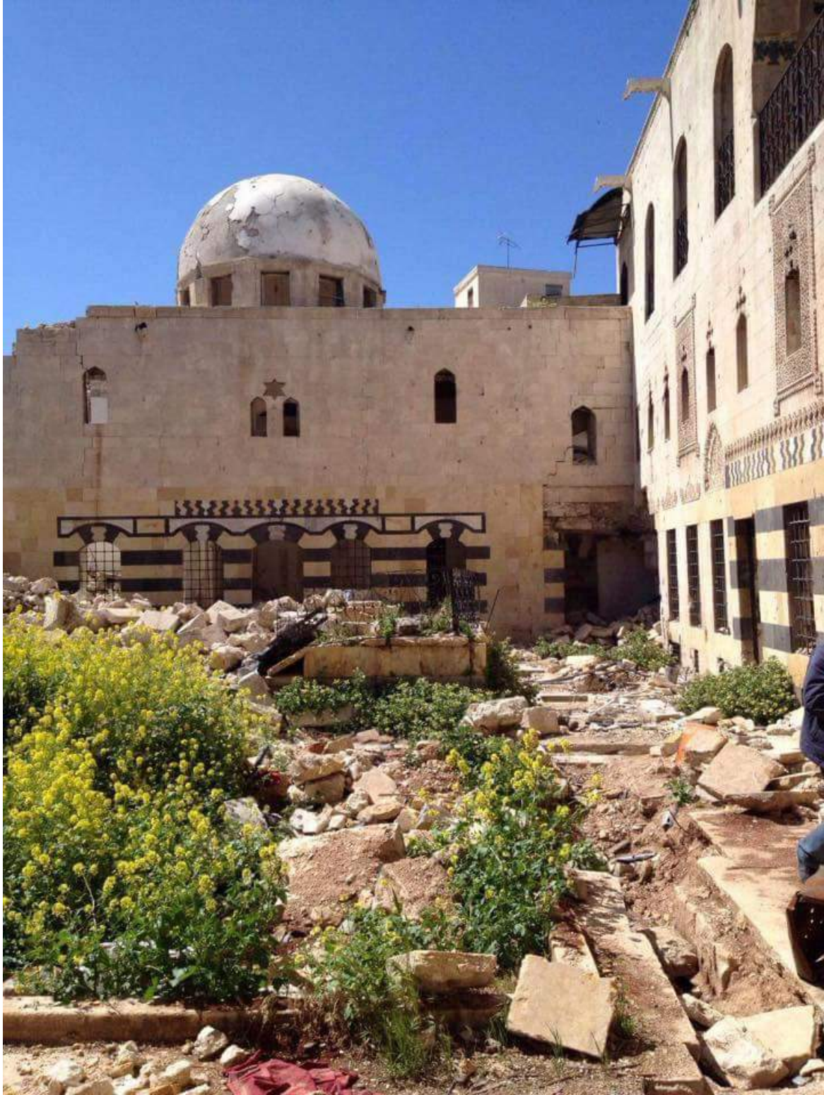
Damage seen inside Beit Ghazaleh (Aleppo Glory; April 3, 2017)
