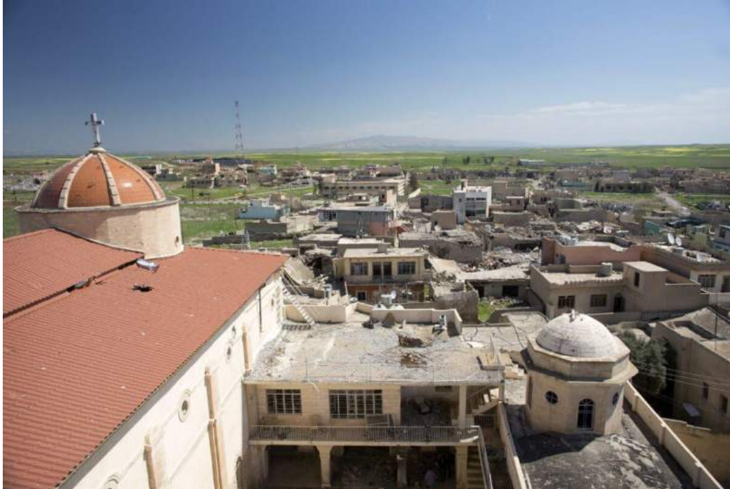
An overhead view of Mar Qoryaqos Church showing some damage to the roof and courtyard (The Ferret; April 13, 2017)
