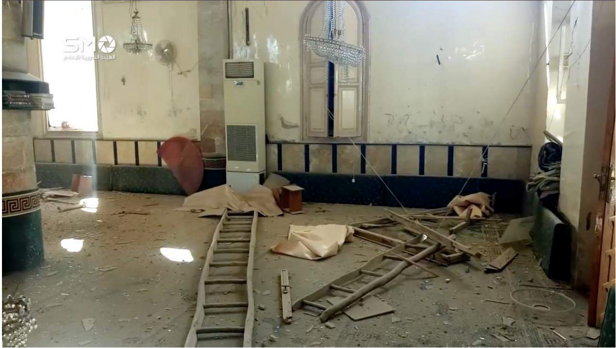
Video still of damage to the interior of Arbin al-Kabir Mosque (SMO Syria; April 8, 2017)
