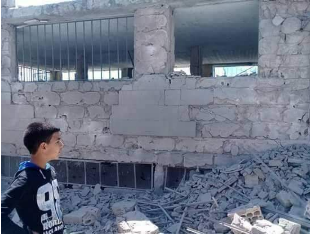
Damage to al-Kabir Mosque (SNHR; April 24, 2017)
