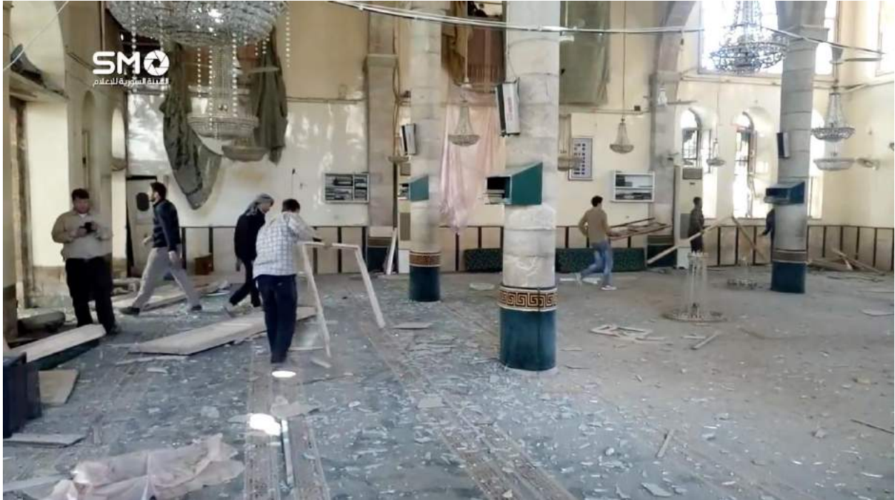
Video still of damage to the interior of Arbin al-Kabir Mosque (SMO Syria; April 8, 2017)
