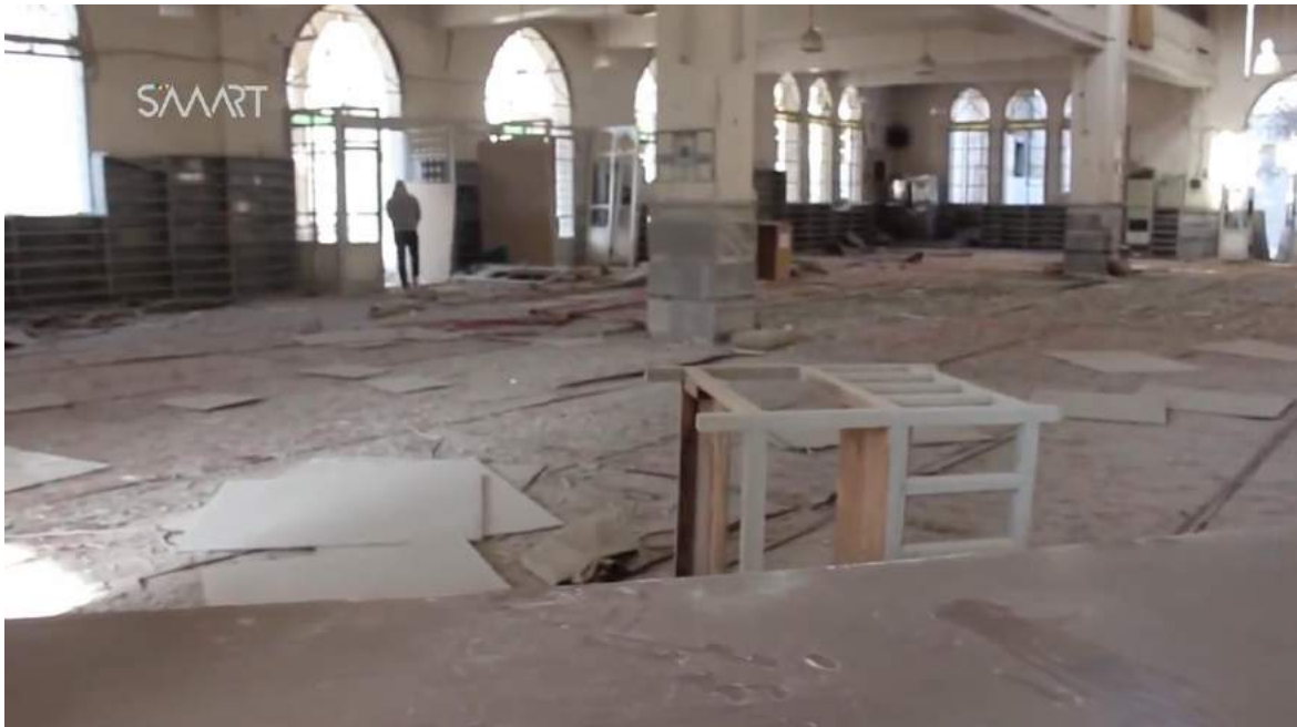
Video still shows damage to the interior of al-Rawda Mosque (Salqin City Coordination; April 7, 2017)
