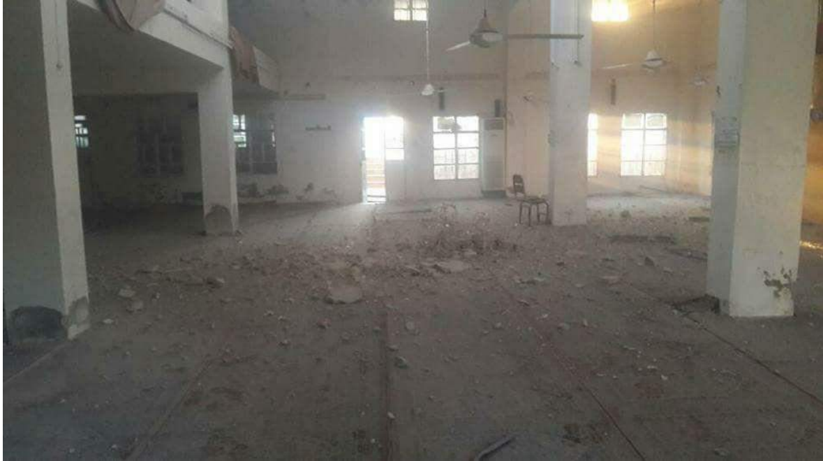
Damage to the interior of Musaib bin Amir Mosque (SNHR; April 25, 2017)
