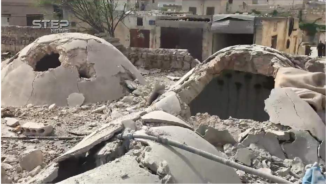
Video still of severe damage to Hammam al-Daraj al-Qadim (Step News Agency; April 27, 2017)
