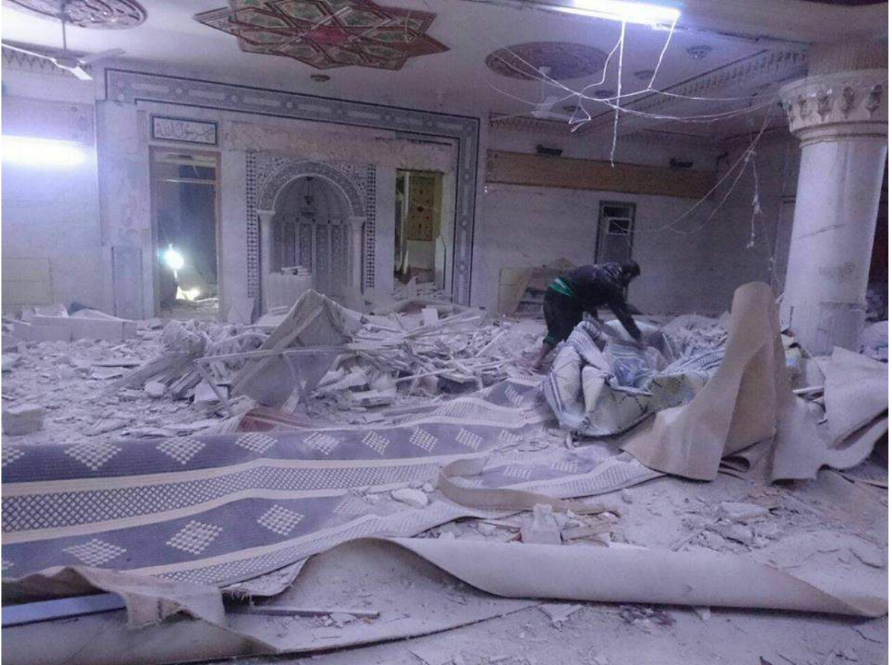
Damage to the interior of the mosque (al-Hal; April 12, 2017)
