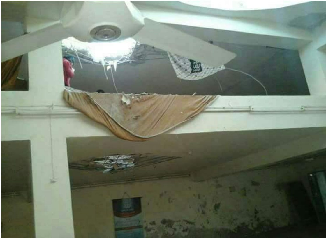
Damage to the interior of Musaib bin Amir Mosque (SNHR; May 9, 2017)
