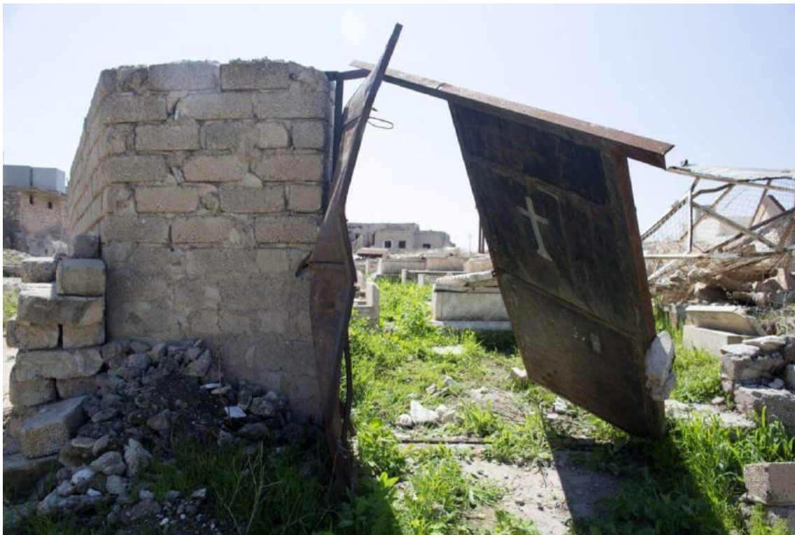
Damage to the Christian Cemetery in Batnaya (The Ferret; April 13, 2017)
