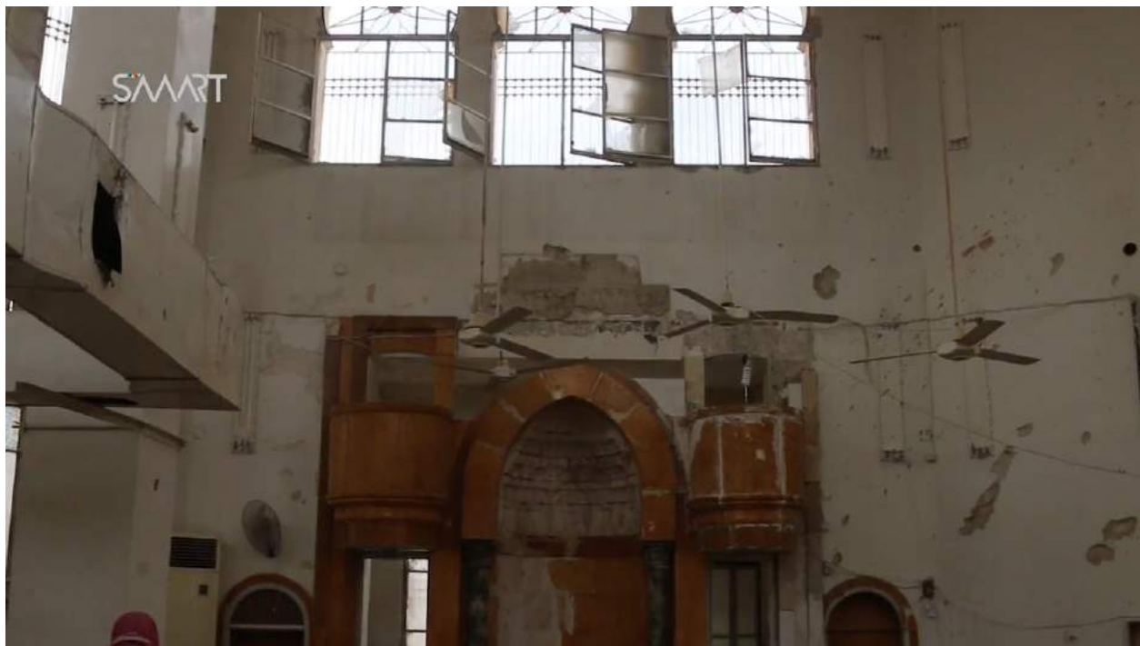
Video still of damage to the interior of Zamzam Mosque (Step News Agency; April 14, 2017)
