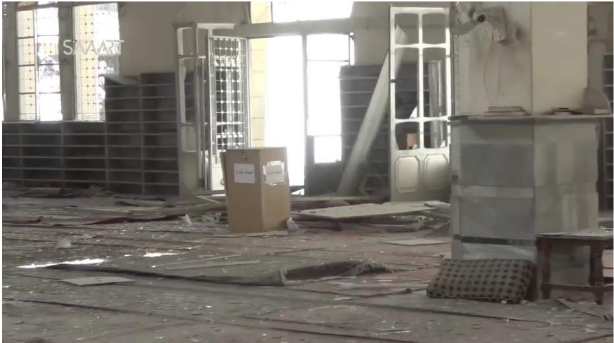
Video still shows damage to the interior of al-Rawda Mosque (Salqin City Coordination; April 7, 2017)
