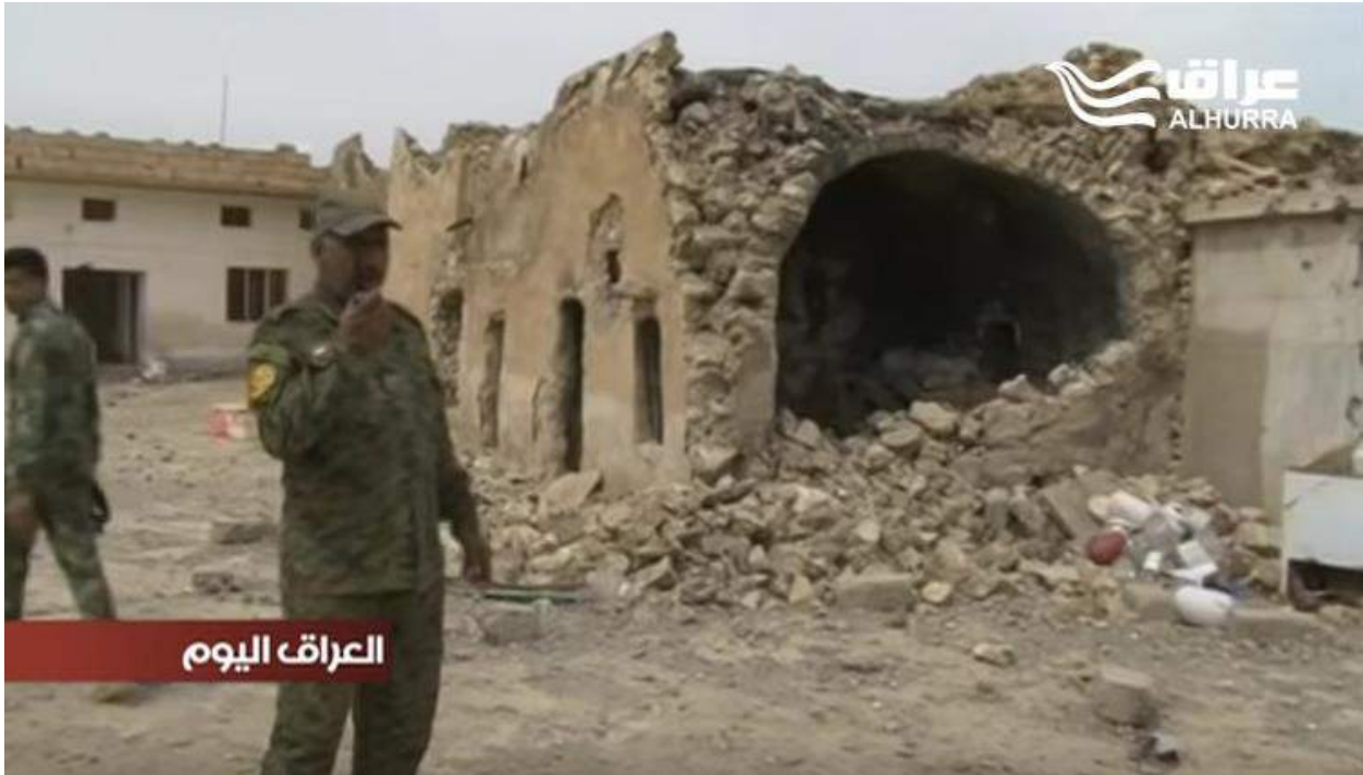
Video still of the village mosque showing evidence of explosives damage (al-Hurra Iraq; April 13, 2017)
