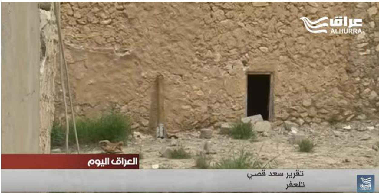
Video still of the village mosque showing evidence of damage and militarization (al-Hurra Iraq; April 13, 2017)
