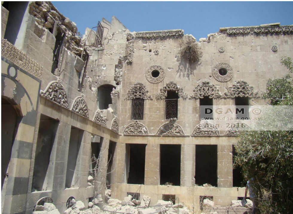
Damage in Beit Ashiqbash courtyard, looking northwest (DGAM; August 20, 2016)
