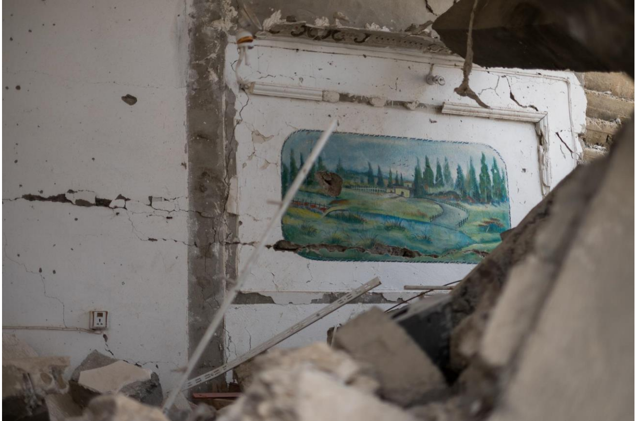
Damage to a wall in an adjoining chapel of the Church of King Jesus (Courtesy of the Preemptive Love Coalition; February 25, 2016)
