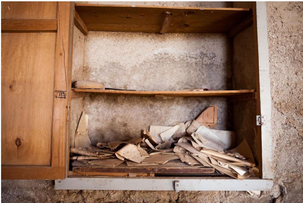
Damage to religious material inside the Church of King Jesus (Courtesy of Preemptive Love Coalition; March 30, 2016)
