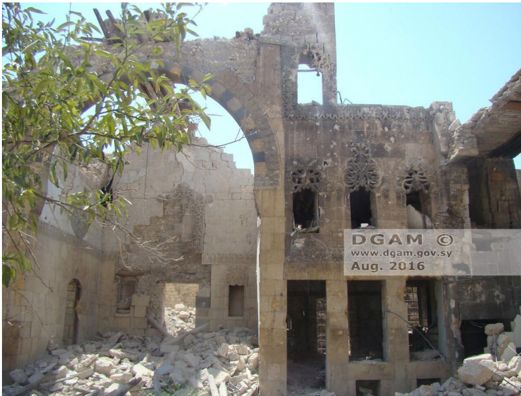
Severe damage to interior courtyard of Beit Ashiqbash, looking south (DGAM; August 20, 2016)
