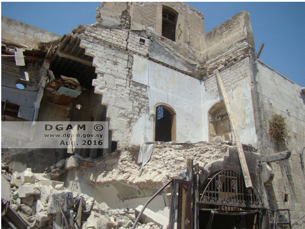
Severe damage to Beit Ghazaleh (DGAM; August 20, 2016)
