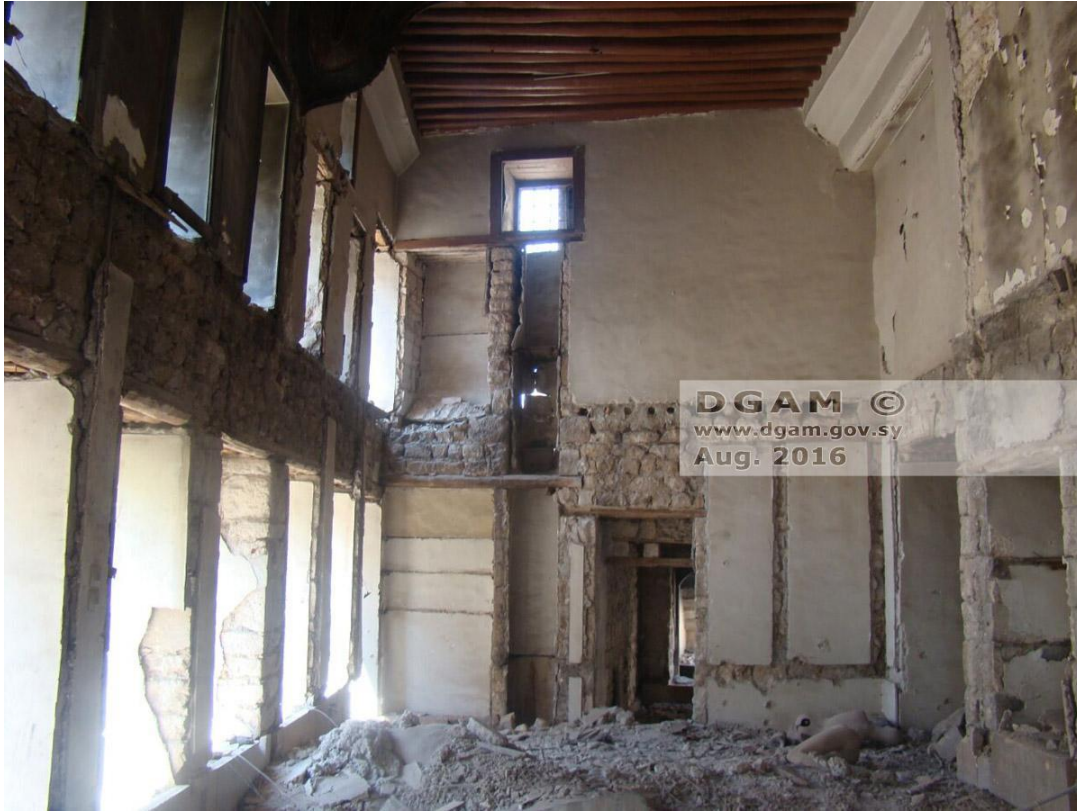
Severe damage to interior of Beit Ashiqbash (DGAM; August 20, 2016)
