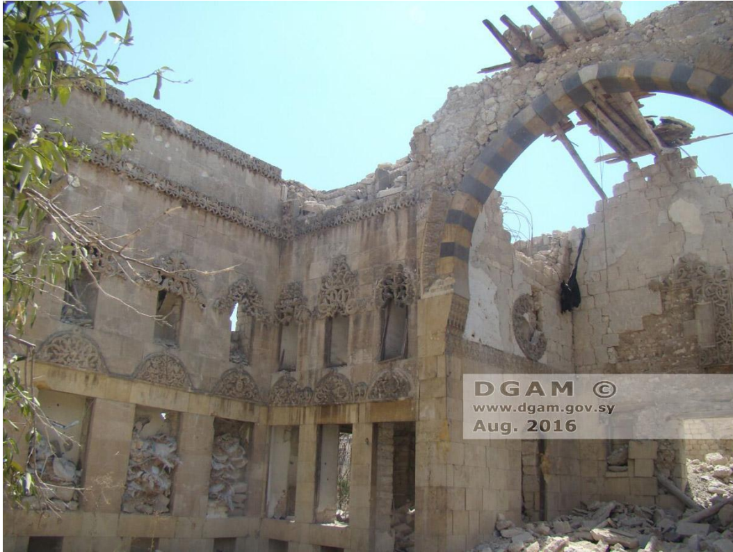
Severe damage to interior courtyard of Beit Ashiqbash, looking southeast (DGAM; August 20, 2016)
