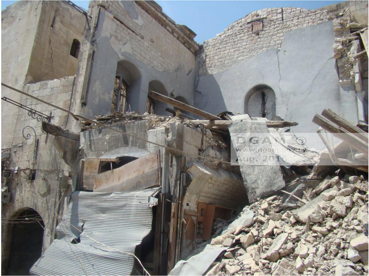
Severe damage to Beit Ghazaleh (DGAM; August 20, 2016)
