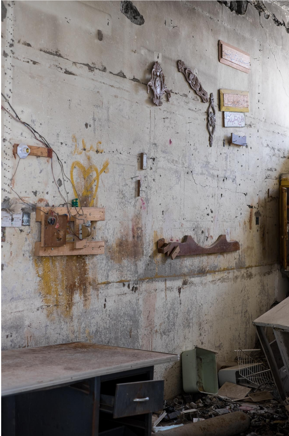
Damage to a wall in an adjoining chapel at the Church of King Jesus (Courtesy of the Preemptive Love Coalition; February 25, 2016)
