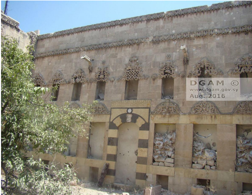
Damage to eastern wall of Beit Ashiqbash courtyard (DGAM; August 20, 2016)
