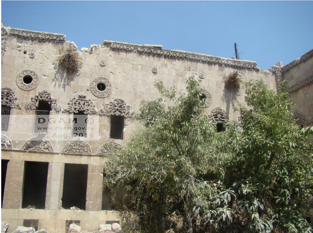
Damage in Beit Ashiqbash courtyard, looking north (DGAM; August 20, 2016)
