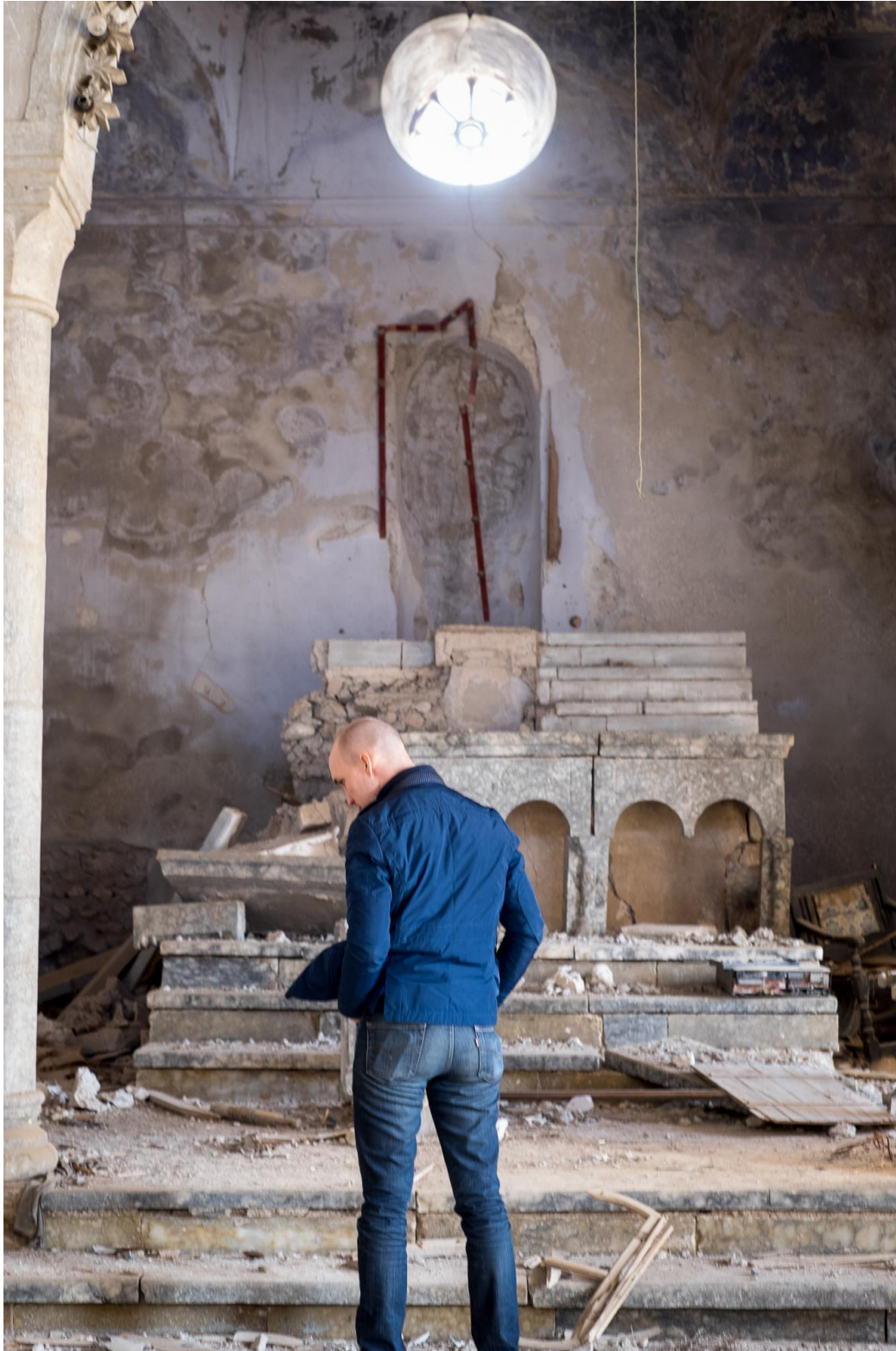
The CEO of the Preemptive Love Coalition observes the damage to the Church of King Jesus (Courtesy of Preemptive Love Coalition; March 30, 2016)
