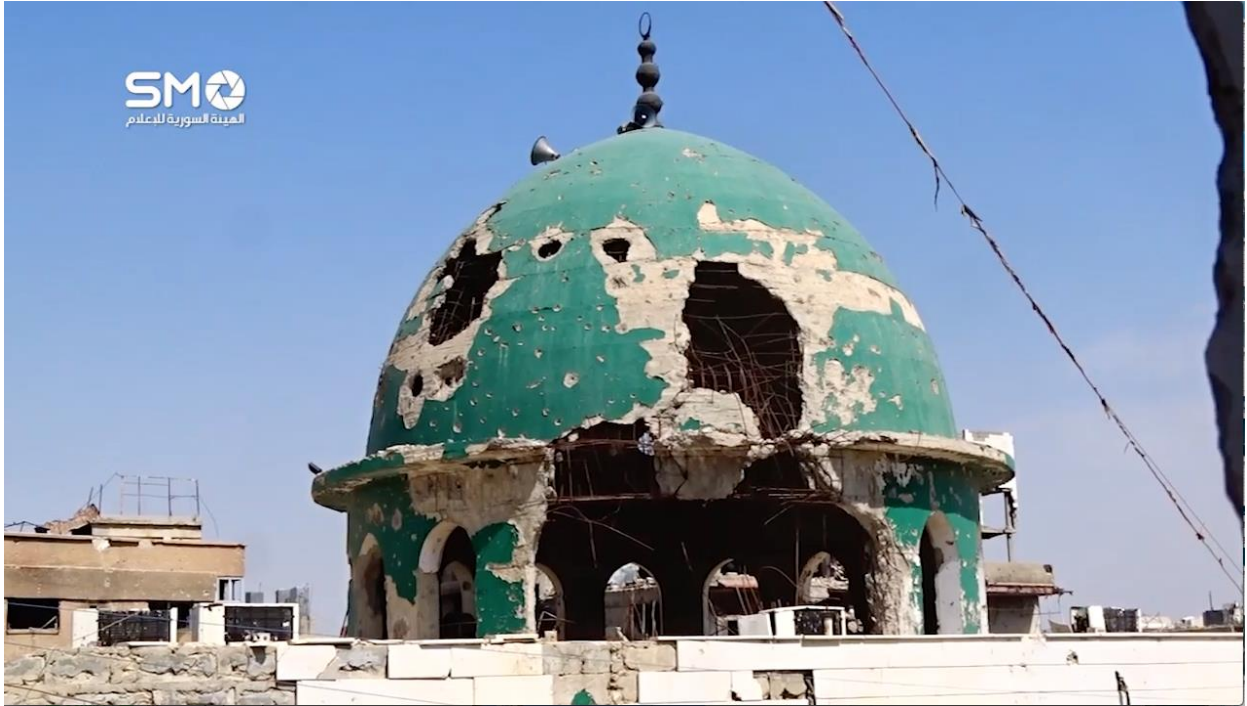
Video still of severe damage to the dome of what is most likely al-Sahaba Abu Bakr al-Sedeiq Mosque (SMO Syria; August 24, 2016)
