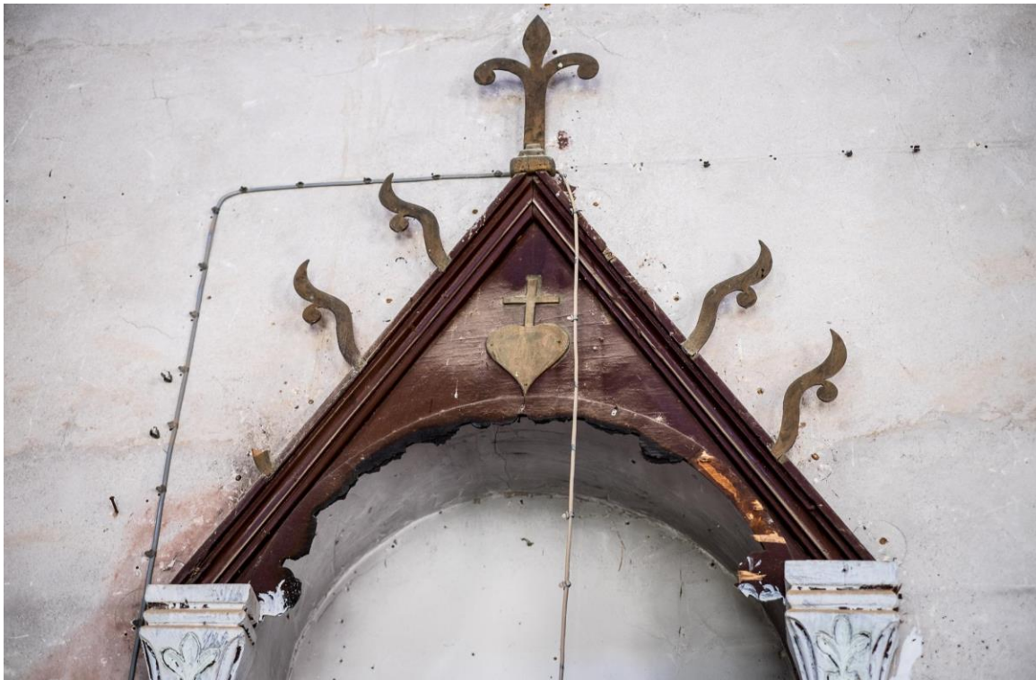
Damage to religious material inside the Church of King Jesus (Courtesy of Preemptive Love Coalition; March 30, 2016)
