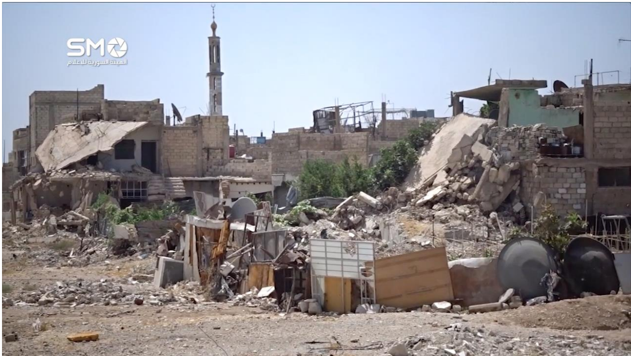
Video still of the damage to the minaret of an unidentified mosque (SMO Syria; August 24, 2016)
