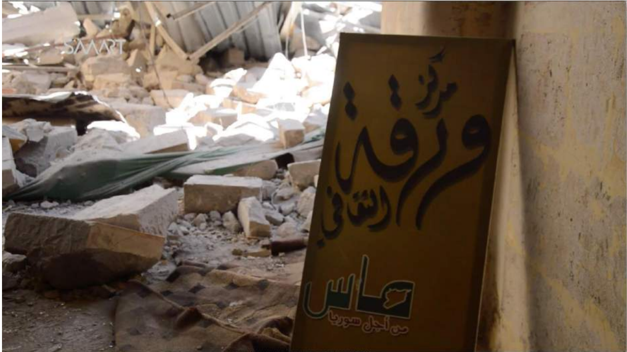
Video still closeup of damage to Waraqa Cultural Center (SMART News Agency; August 15, 2016)
