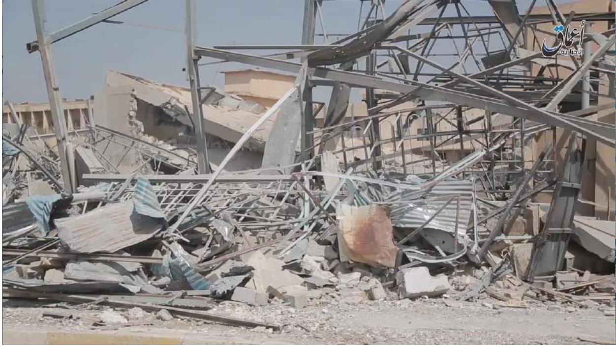
Video still of damage to the Faculty of Science (Amaq News Agency/Youtube; August 6, 2016)
