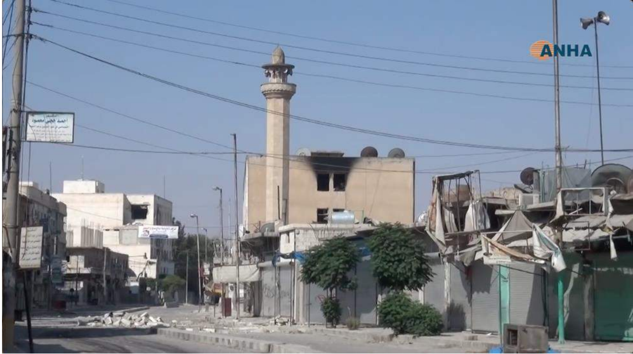
Video still of the minaret of al-Kabir Mosque showing no damage (ANHA; August 11, 2016)
