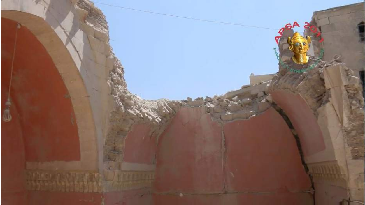
Video still of detail of the damage to Waraqa Cultural Center (APSA; August 16, 2016)
