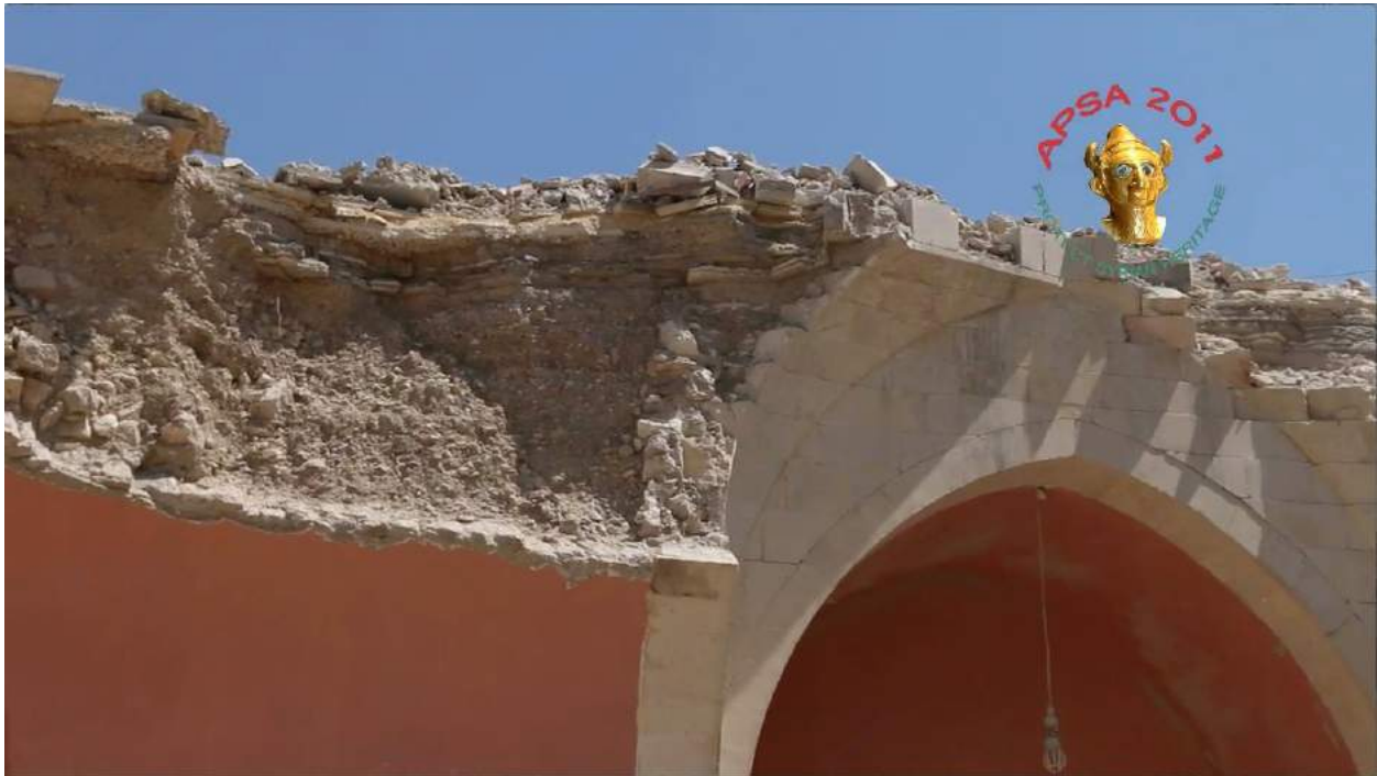
Video still of detail of the damage to Waraqa Cultural Center (APSA; August 16, 2016)
