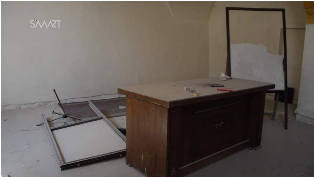
Video still of damage to a classroom at Waraqa Cultural Center (SMART News Agency; August 15, 2016)
