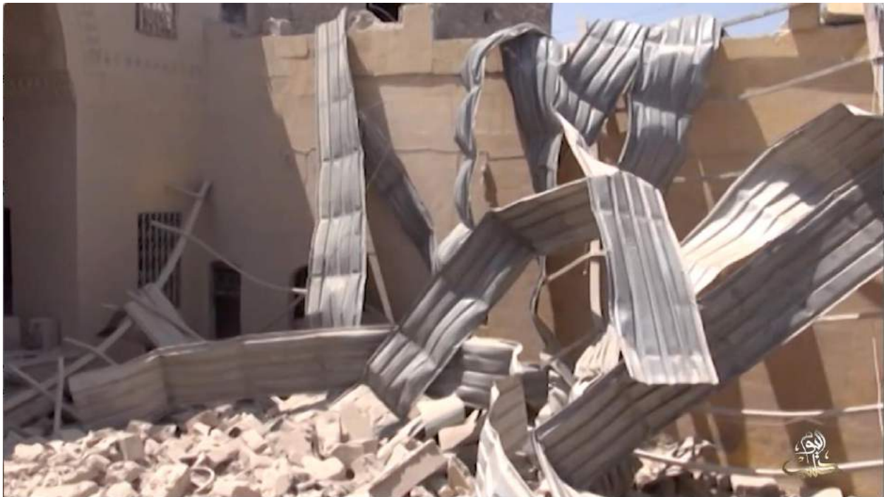
Video still of damage to a room of Waraqa Cultural Center, showing the collapse of the entire ceiling (Halab Today TV; August 15, 2016)
