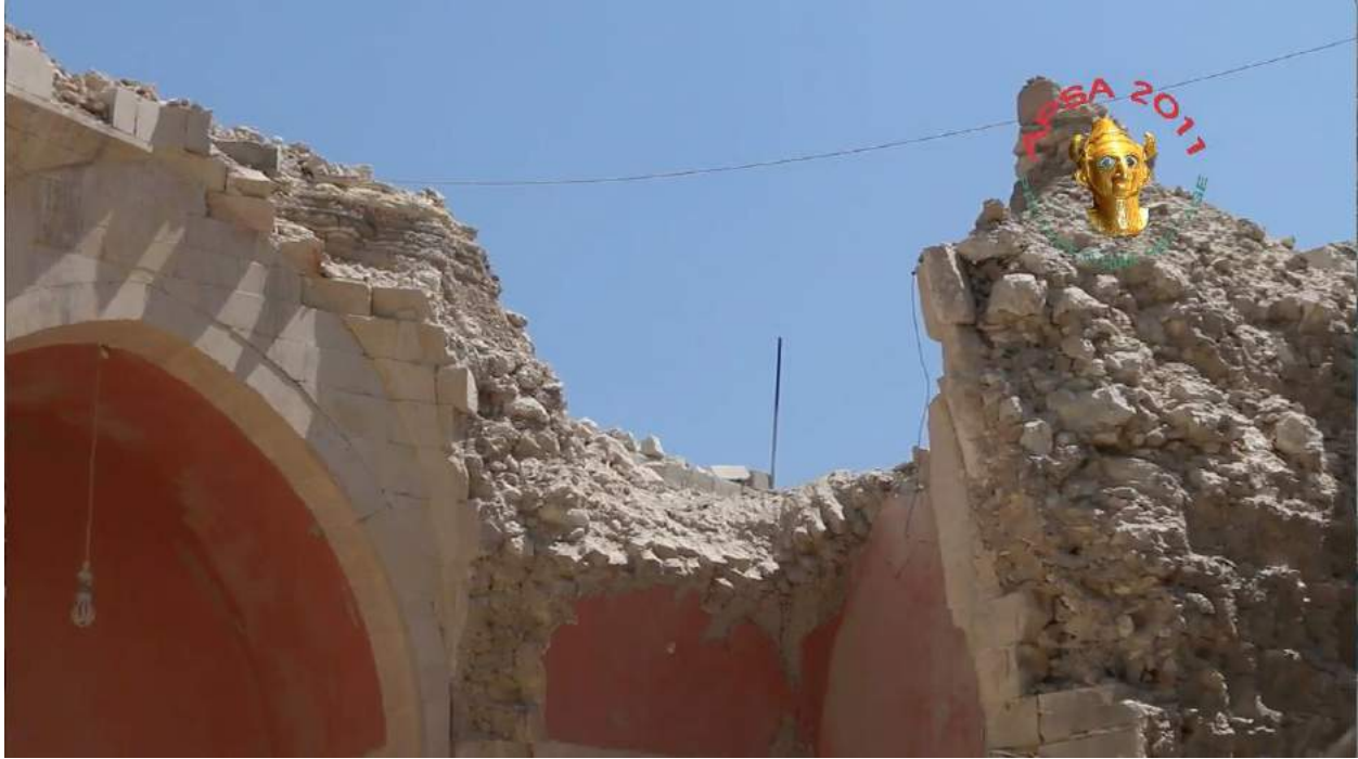
Video still of detail of the damage to Waraqa Cultural Center (APSA; August 16, 2016)
