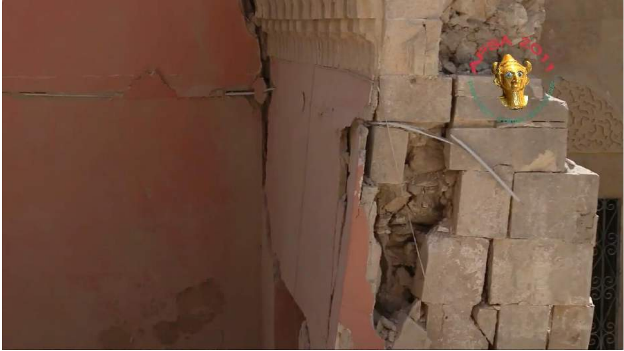
Video still of detail of the damage to Waraqa Cultural Center (APSA; August 16, 2016)
