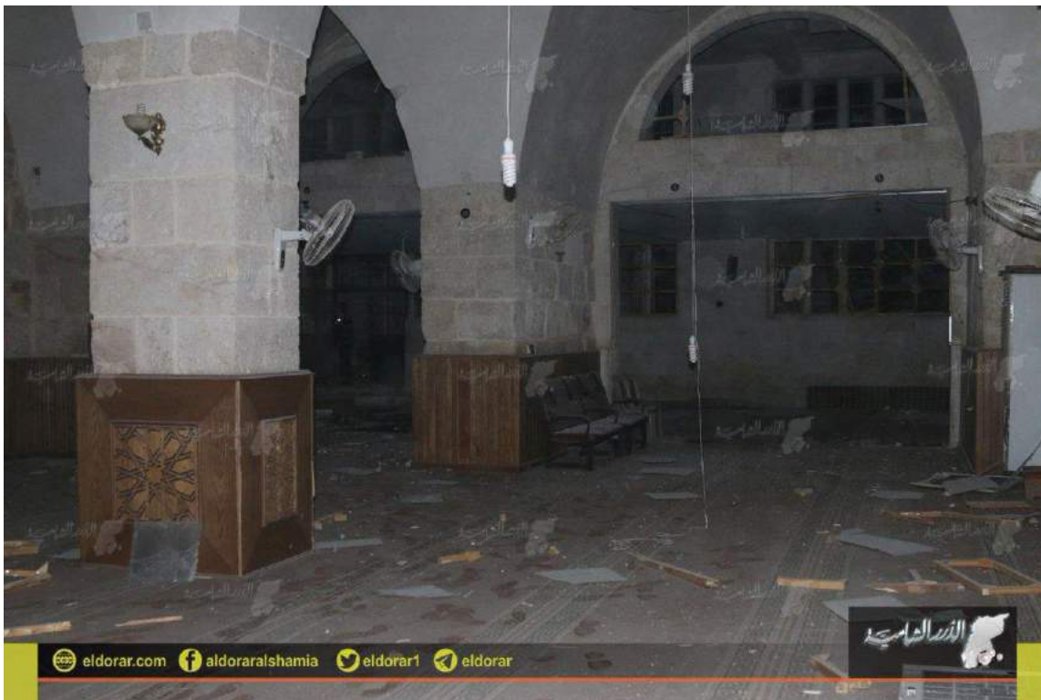
Interior damage to al-Kabir Mosque (Al Dorar Al Shamia; August 8, 2016)
