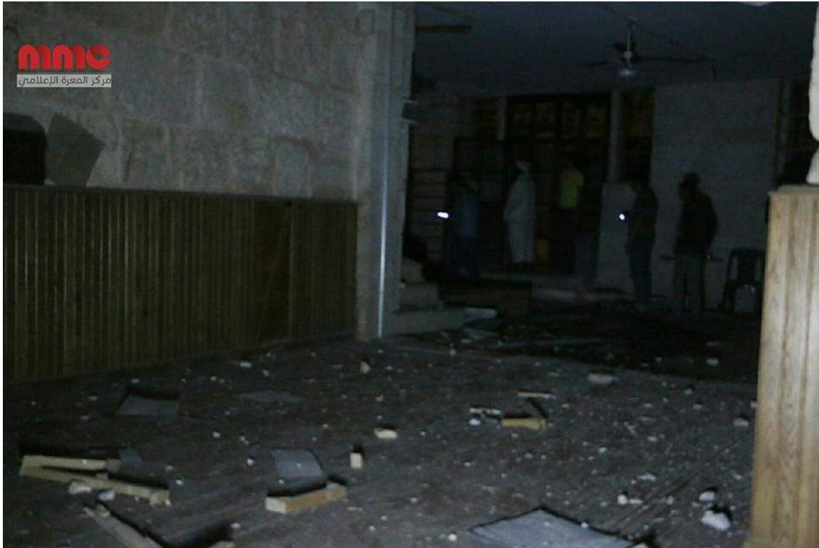
Interior damage to al-Kabir Mosque (SNHR; August 8, 2016)
