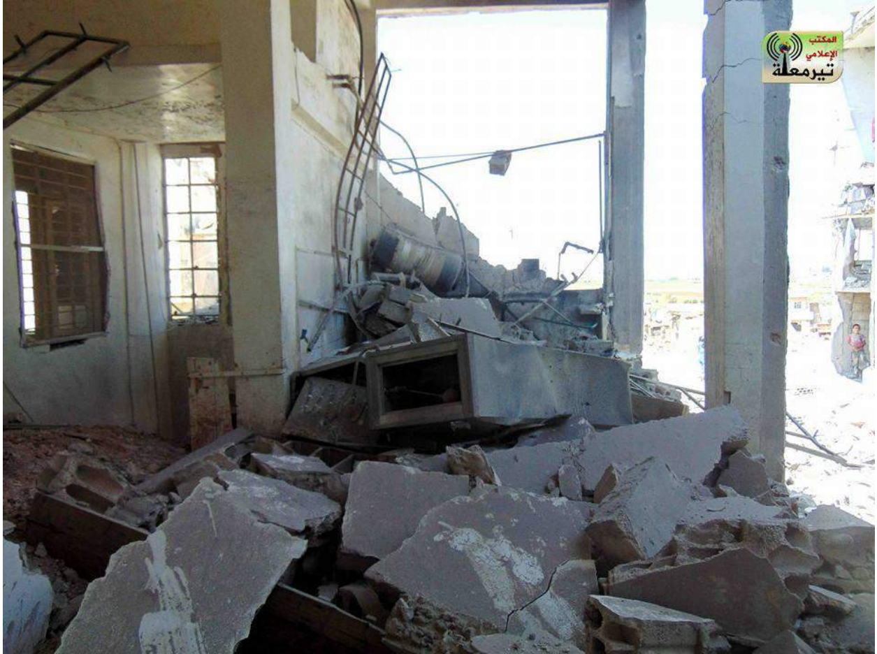
Damage to Abu Bakr al-Sedeiq Mosque (SNHR; August 12, 2016)
