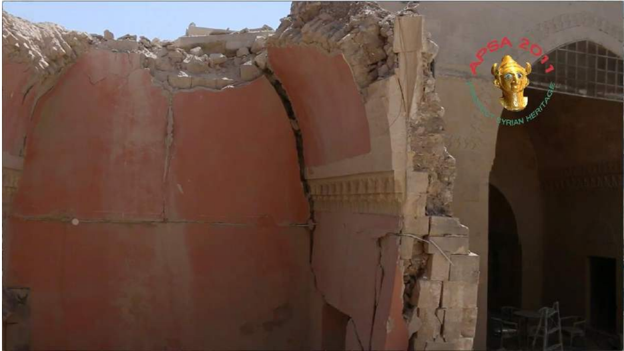
Video still of detail of the damage to Waraqa Cultural Center (APSA; August 16, 2016)
