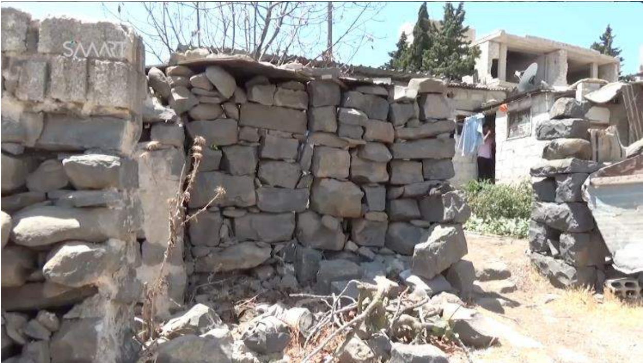
Video still of Byzantine structures reused by modern inhabitants (SMART News Agency; August 11, 2016)
