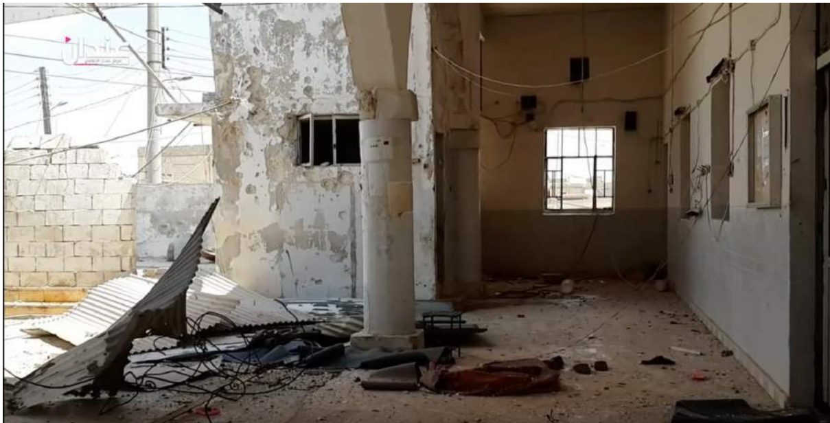
Video still of damage to the interior and courtyard of al-Kabir Mosque (Anadan Media Center; August 13, 2016)
