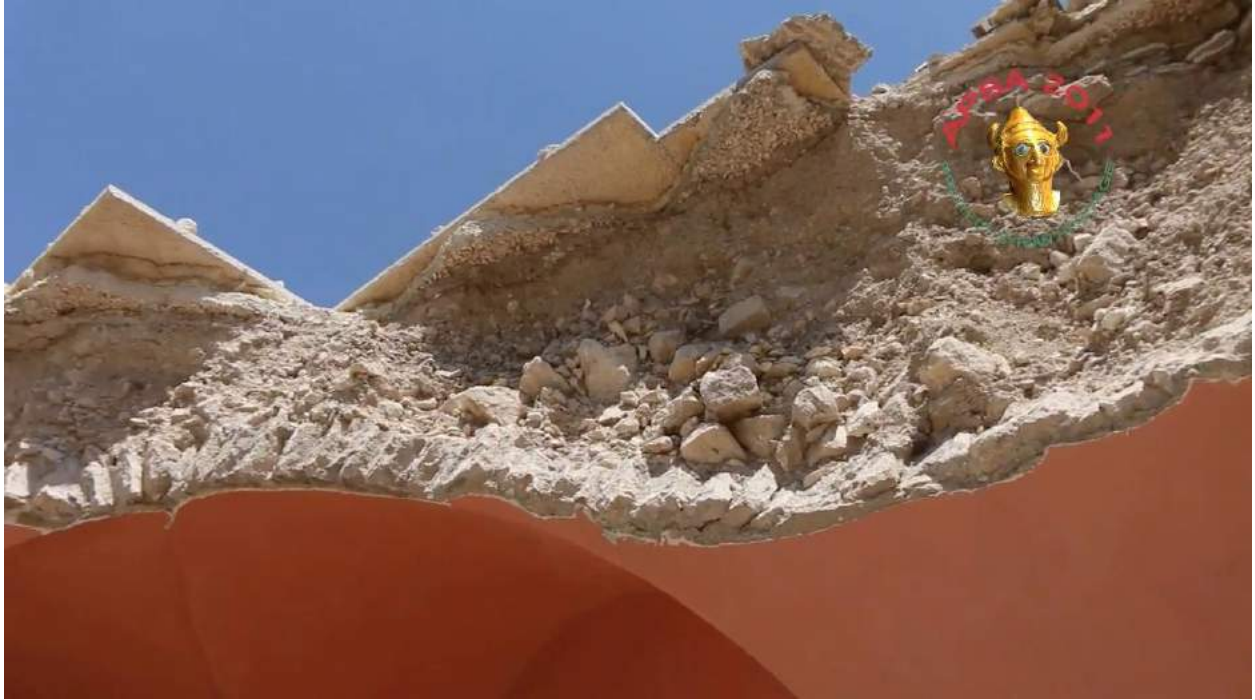
Video still of detail of the damage to Waraqa Cultural Center (APSA; August 16, 2016)
