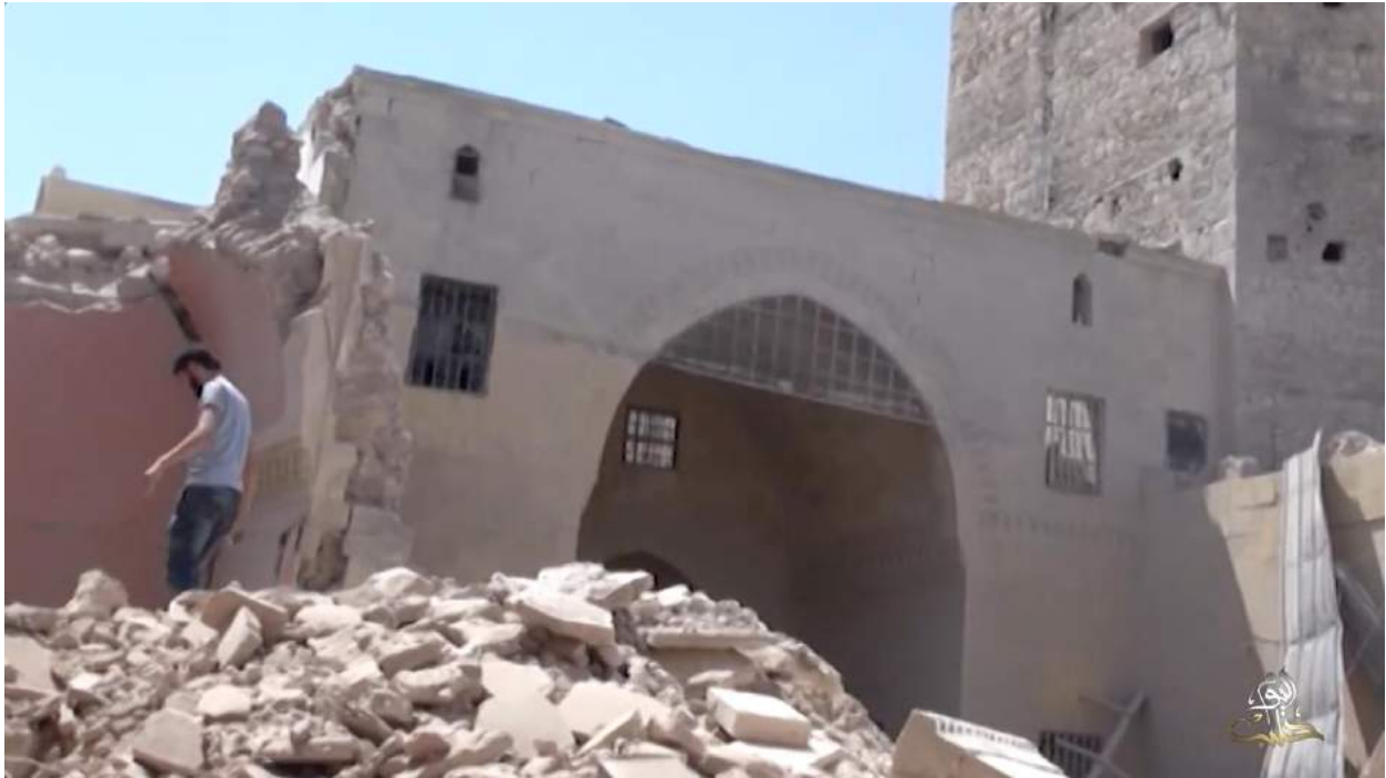
Video still of extensive damage to Waraqa Cultural Center (Halab Today TV; August 15, 2016)
