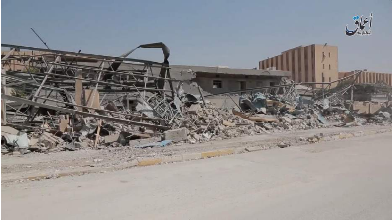
Video still of damage to the Faculty of Science (Amaq News Agency/Youtube; August 6, 2016)
