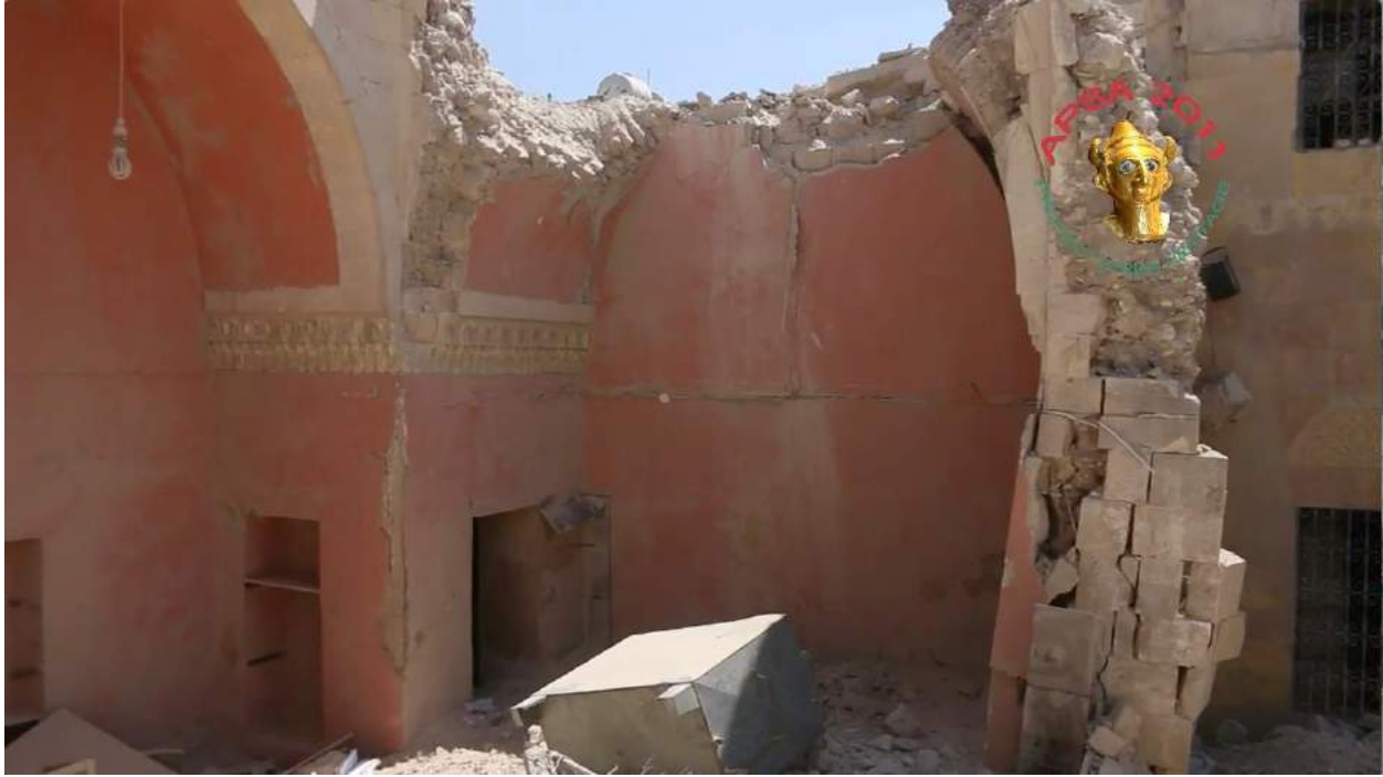
Video still of damage to Waraqa Cultural Center (APSA; August 16, 2016)
