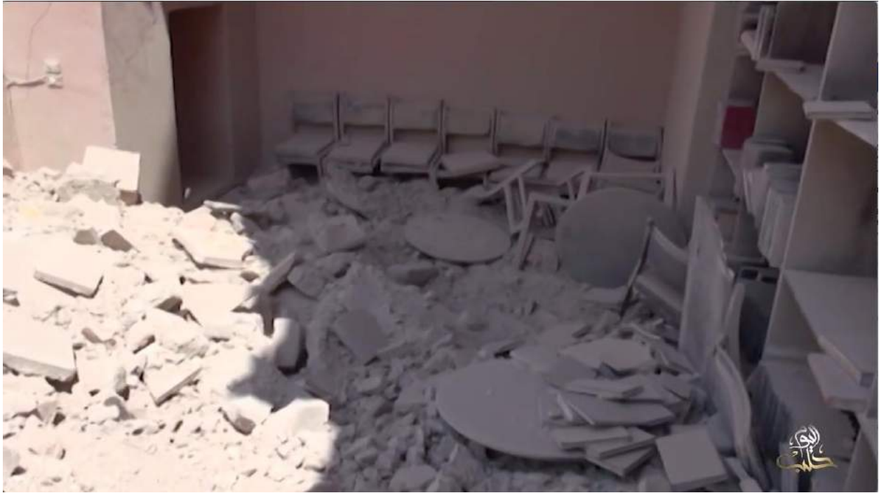
Video still of material damage at Waraqa Cultural Center (Halab Today TV; August 15, 2016)
