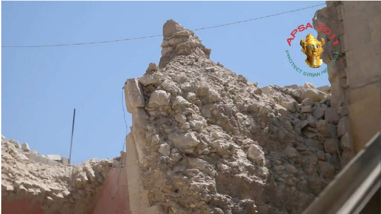
Video still of detail of the damage to the Waraqa Cultural Center (APSA; August 16, 2016)
