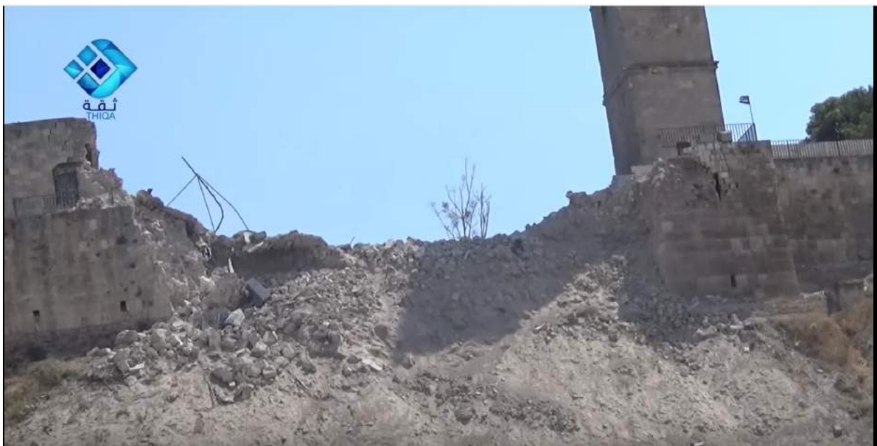
Video still of the damage to the northern side of the Citadel of Aleppo, with the Citadel Museum on the left (Thiqa News Agency; August 11, 2016)
