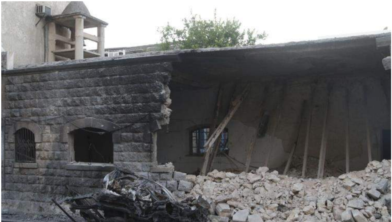
Damage to the church showing a collapsed wall and ceiling beams (Baladi News; August 13, 2016)
