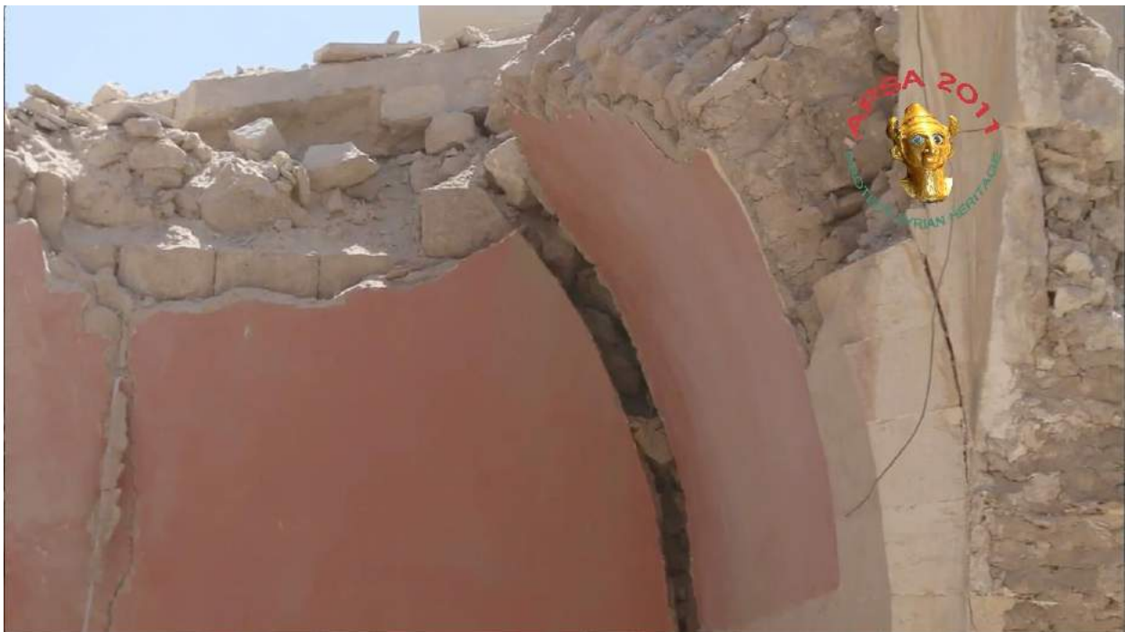
Video still of detail of the damage to Waraqa Cultural Center (APSA; August 16, 2016)
