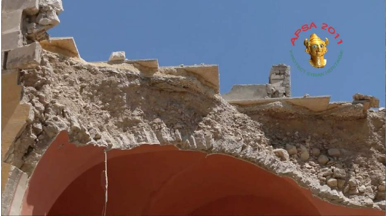
Video still of detail of the damage to Waraqa Cultural Center (APSA; August 16, 2016)
