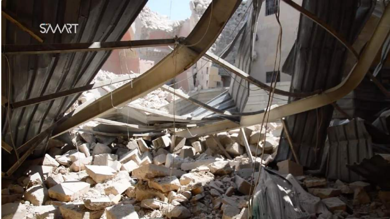
Video still of the collapsed ceiling at Waraqa Cultural Center (SMART News Agency; August 15, 2016)
