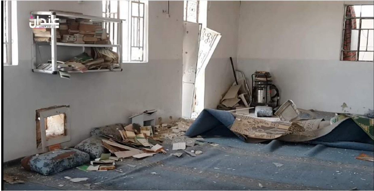
Video still of damage to the interior of al-Kabir Mosque (Anadan Media Center; August 13, 2016)
