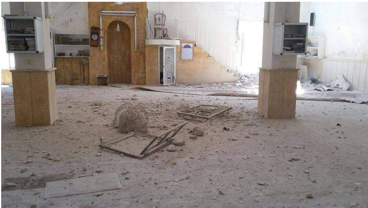
Damage to al-Hassan Mosque (Halab Today TV; August 15, 2016)
