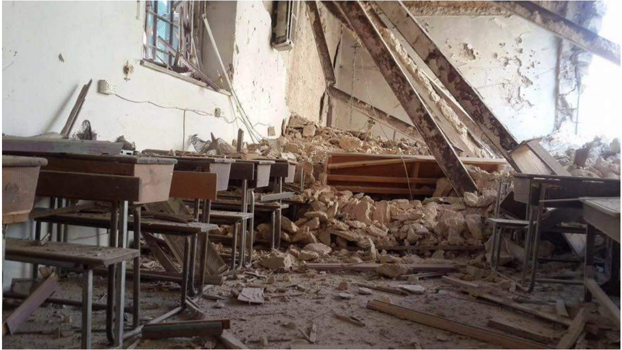
Damage to the classroom located within the church (Facebook; August 10, 2016)
