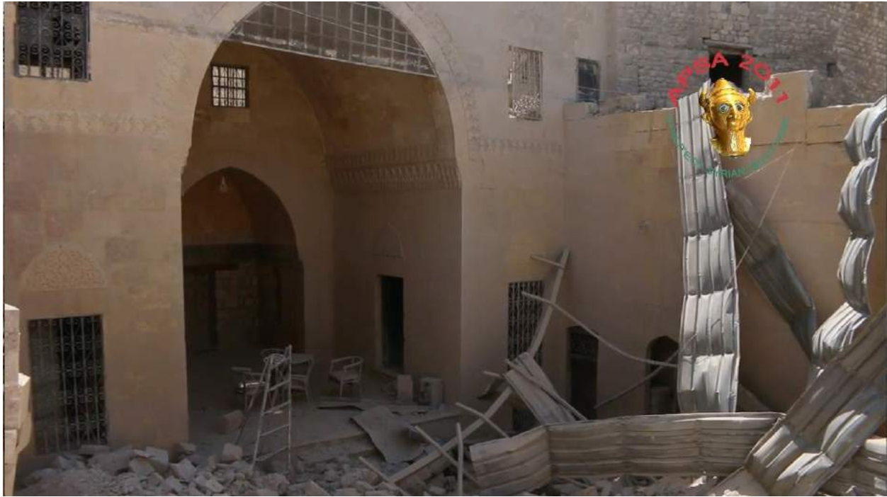
Video still of extensive damage to Waraqa Cultural Center (APSA; August 16, 2016)
