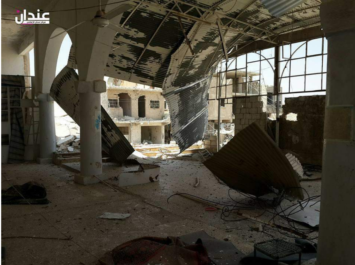
Severe damage to the interior of al-Kabir Mosque (SNHR; August 14, 2016)
