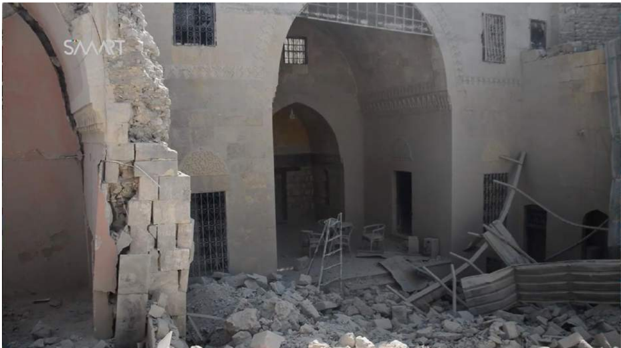
Video still of extensive damage to Waraqa Cultural Center (SMART News Agency; August 15, 2016)
