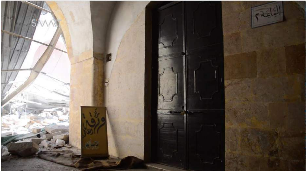
Video still of damage to Waraqa Cultural Center (SMART News Agency; August 15, 2016)
