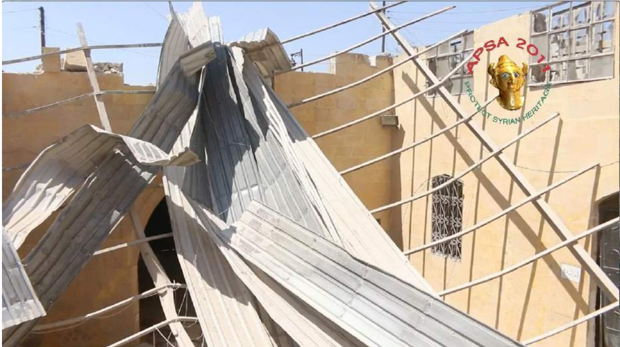
Video still of detail of the damage to the ceiling of Waraqa Cultural Center (APSA; August 16, 2016)
