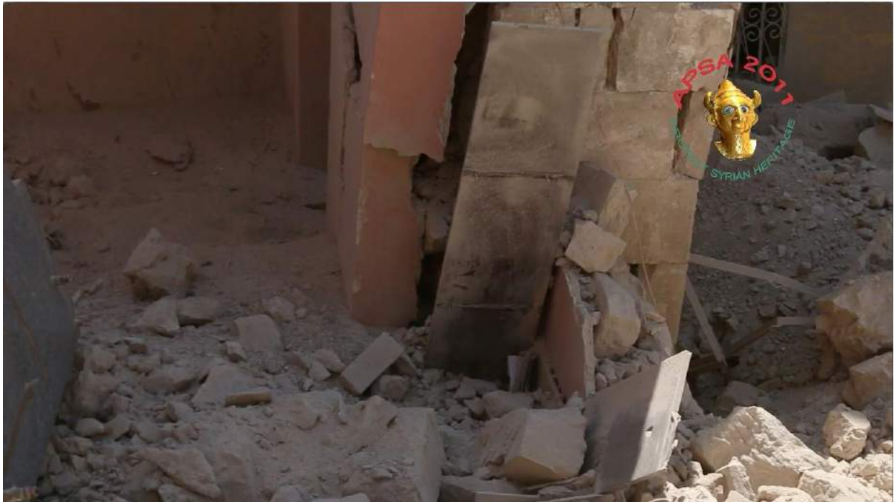
Video still of detail of the damage to Waraqa Cultural Center (APSA; August 16, 2016)
