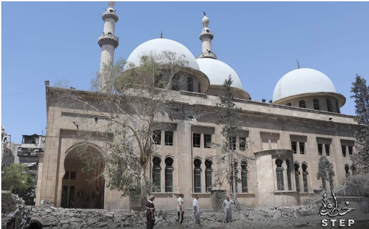
Damage to the exterior of Abdul Qadir Gilani Mosque (Step News Agency/Twitter; July 21, 2016)
