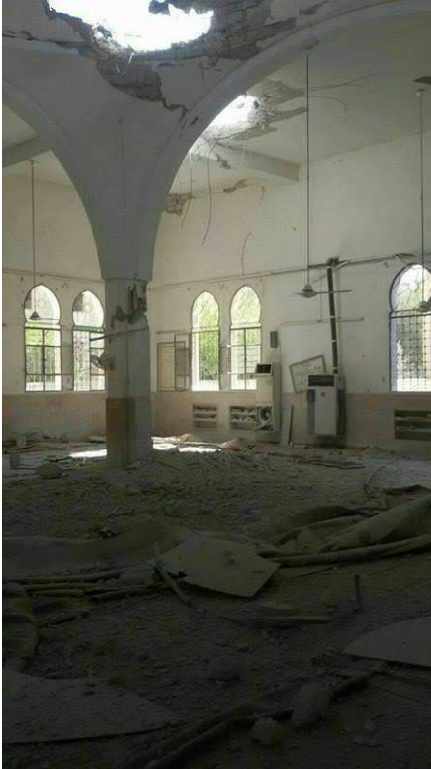
Damage to the interior of al-Rawda Mosque (SNHR; July 19, 2016)
