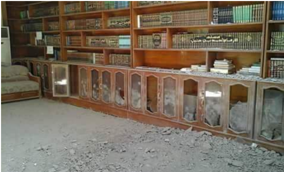
Damage and debris in al-Shamari Mosque library (Fajr al-Iraq News/Twitter; September 21, 2015)
