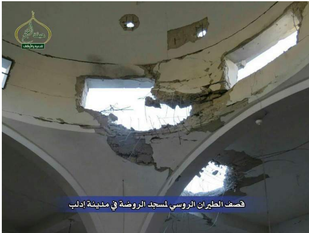
Holes in the dome and walls of al-Rawda Mosque (Committee for Preaching and Endowment; July 19, 2016)
