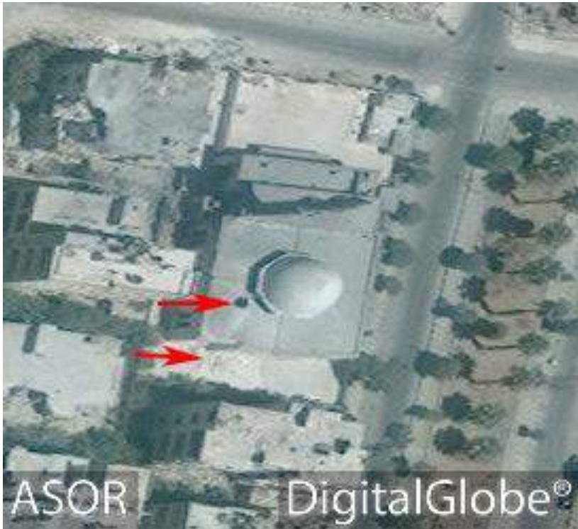
al-Rawda Mosque with damage to the roof and debris seen on the south side (DigitalGlobe; August 1, 2016)
