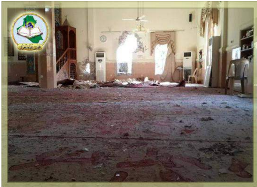
Damage and debris in interior of Hamza Abbas al-Isawi Mosque (Majlis Iraq; August 17, 2014)
