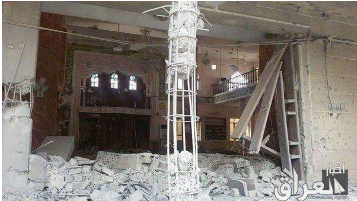
Damage to the outside of Shaker al Dahi Mosque (Twitter; May 31, 2015)
