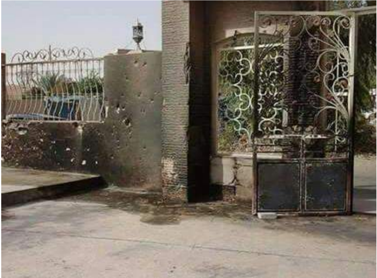
Minor damage to the exterior al-Kabir Mosque (Twitter; September 1, 2015)
