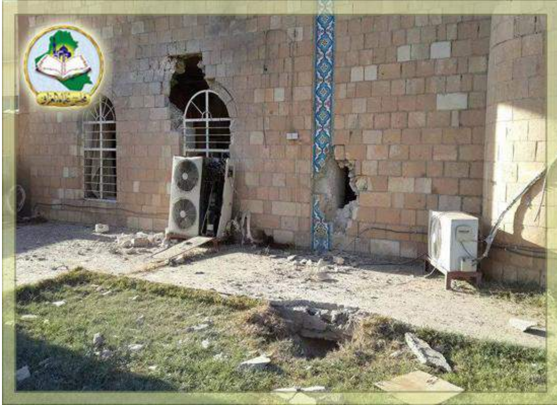
Damage to exterior of Sheikh Hamza Abbas al-Isawi Mosque (Majlis Iraq; August 17, 2014)
