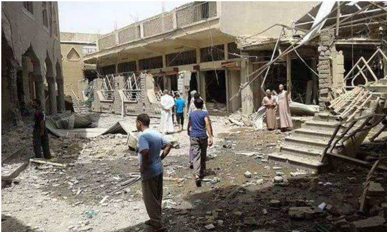
Exterior damage to Shaker al Dahi Mosque (Twitter; May 31, 2015)
