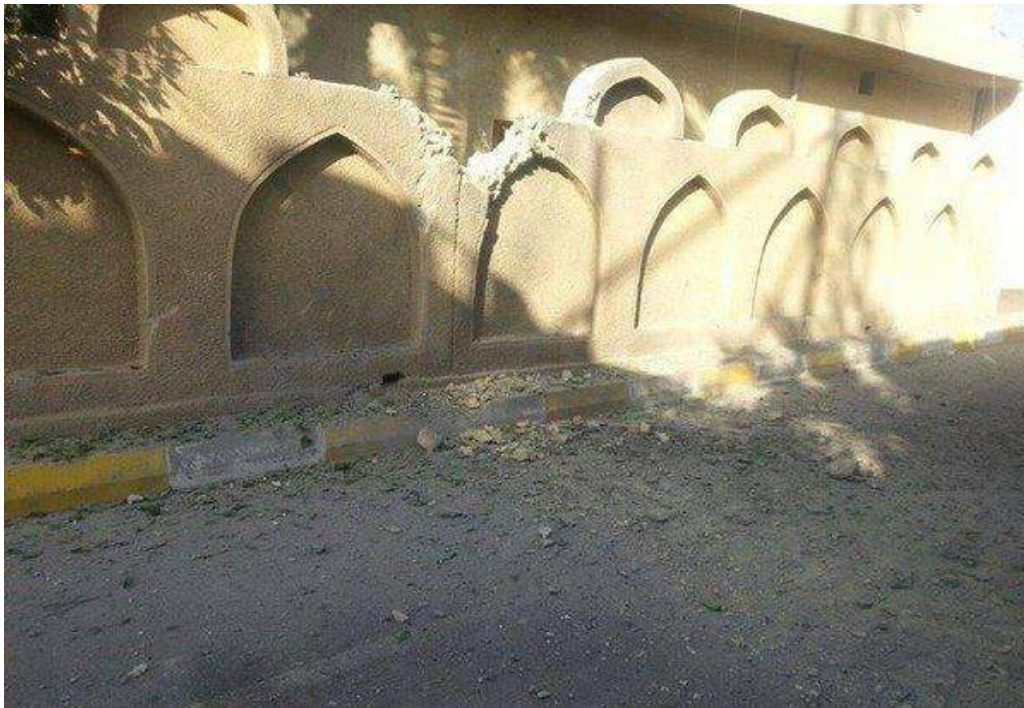
Damage to exterior wall of al-Fayad Mosque (Twitter; November 15, 2014)
