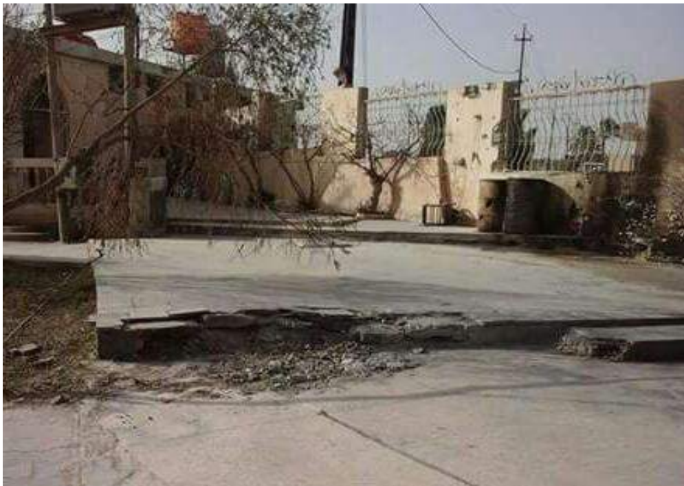
Minor damage to the exterior of al-Kabir Mosque (Twitter; September 1, 2015)
