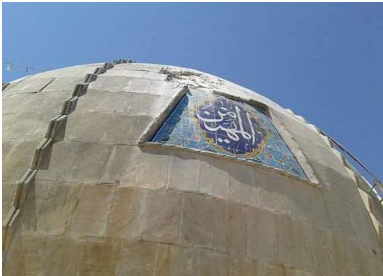
Minor damage to dome on entrance gate to al-Shamari Mosque complex (Twitter; August 10, 2015)
