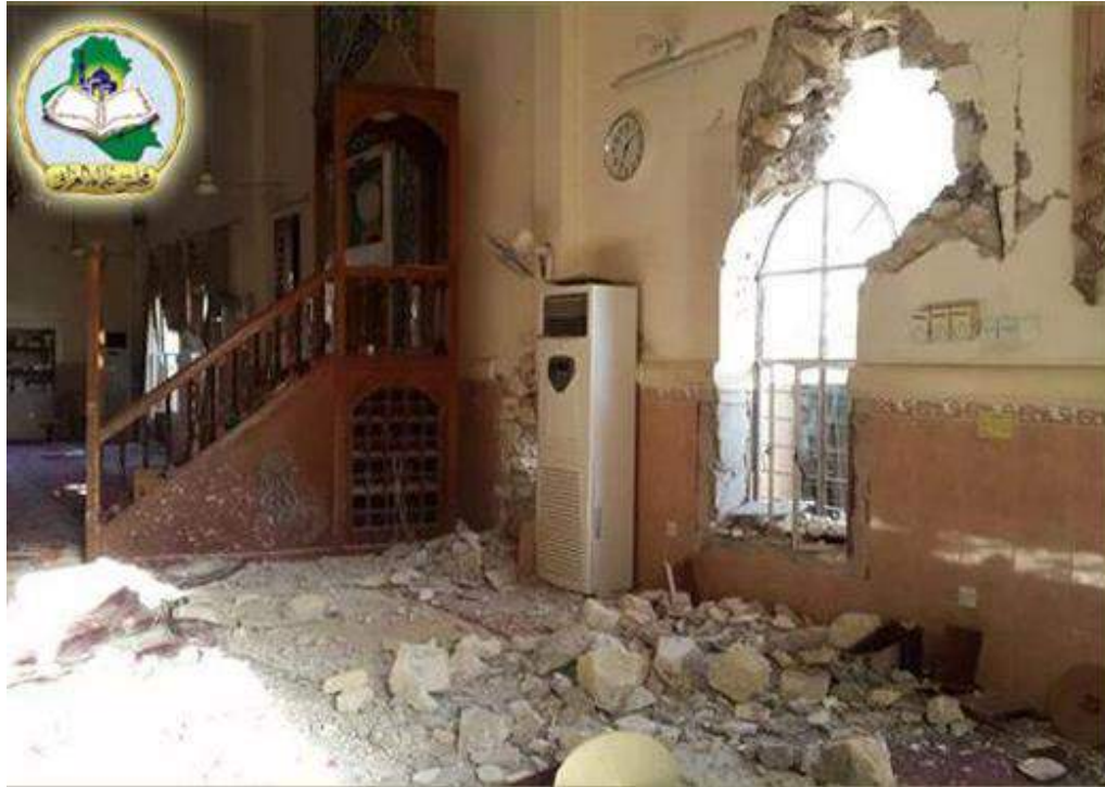
Damage and debris in interior of Hamza Abbas al-Isawi Mosque (Majlis Iraq; August 17, 2014)
