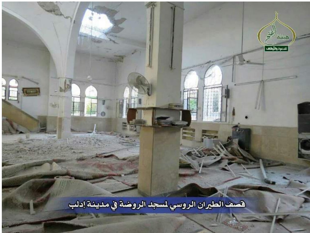
Interior and material damage to al-Rawda Mosque (Committee for Preaching and Endowment; July 19, 2016)
