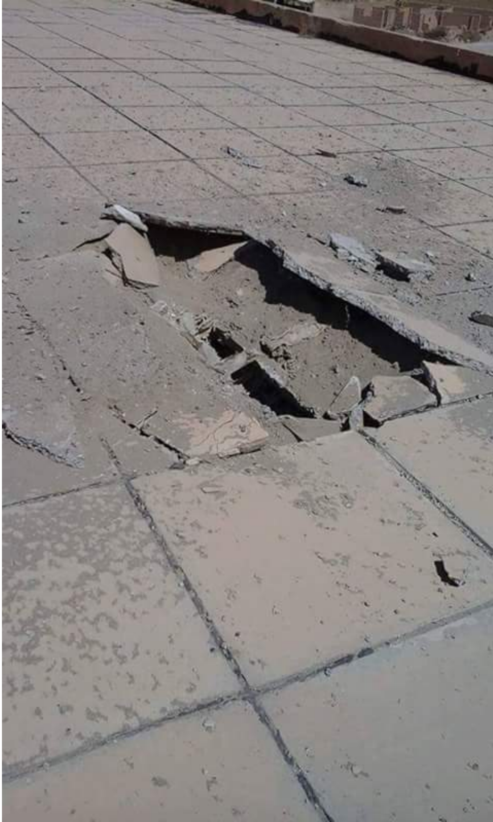
Damage to al-Shamari Mosque courtyard (Fajr al-Iraq News/Twitter; September 21, 2015)
