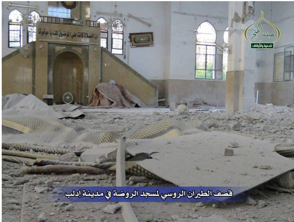
Interior damage to al-Rawda Mosque (Committee for Preaching and Endowment; July 19, 2016)
