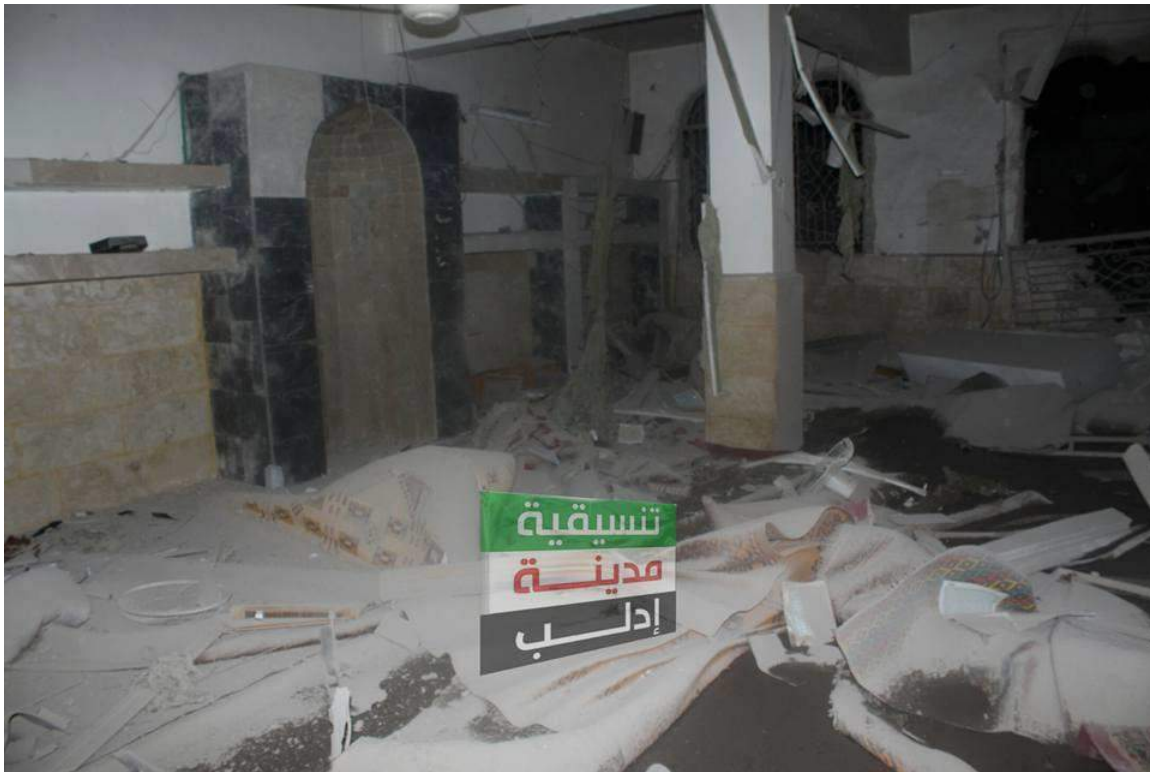
Damage to al-Hijazi Mosque (S.N.N; July 22, 2016)
