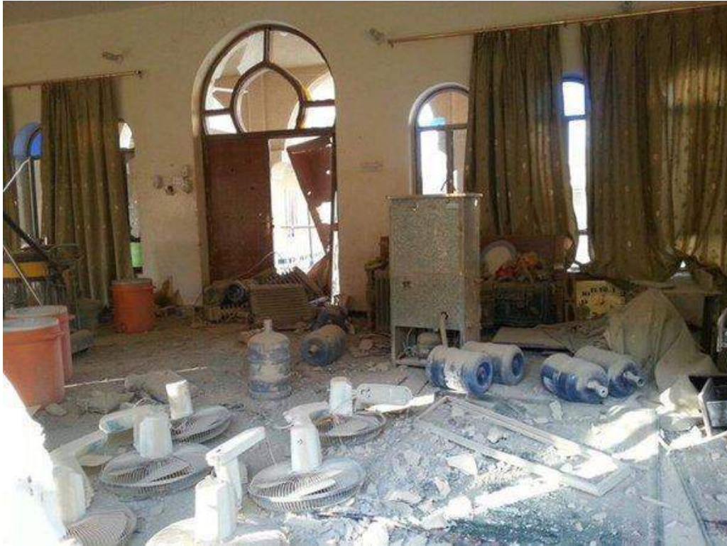
Damage and debris in interior of al-Fayad Mosque (Twitter; November 15, 2014)
