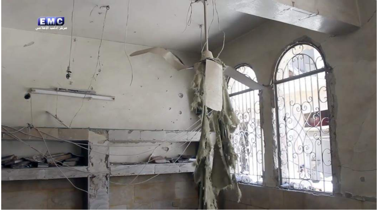
Video still of damage to the ceiling fan and interior of al-Hijazi Mosque (Edlib Media-Center; July 22, 2016)
