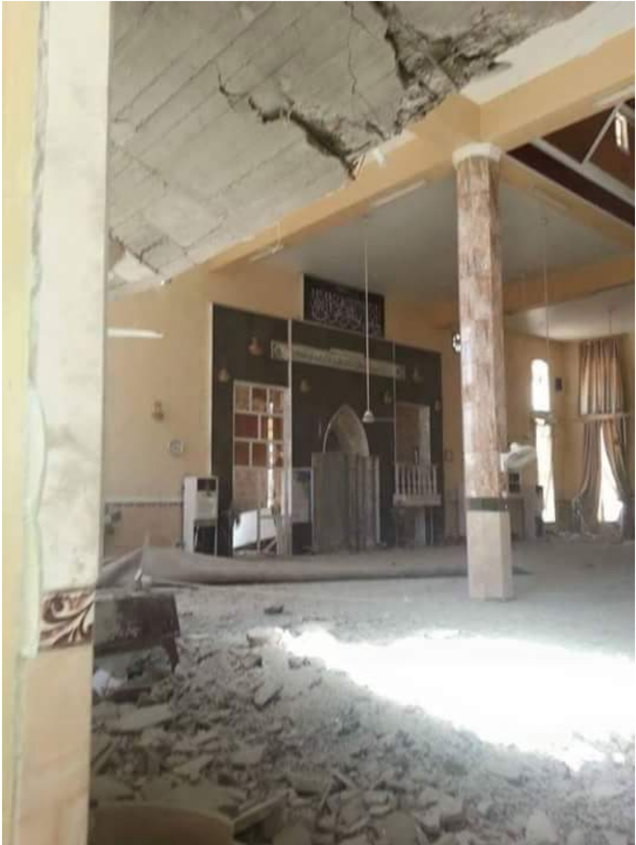
Damage and debris in interior of al-Shamari Mosque (Twitter; August 10, 2015)
