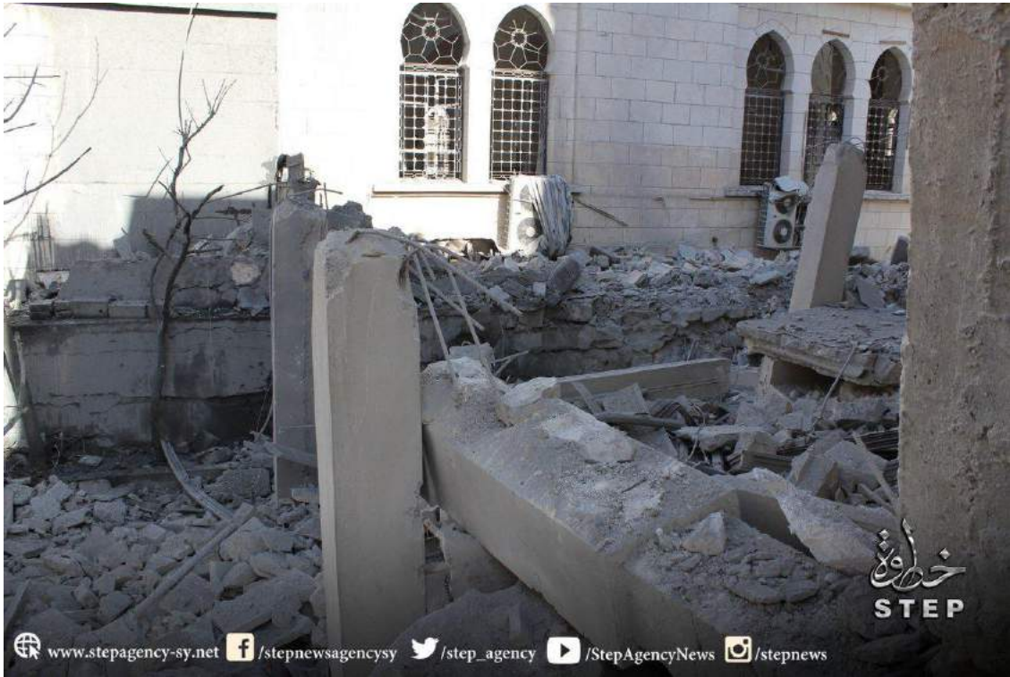
Exterior damage to al-Rawda Mosque (Step News Agency; July 19, 2016)
