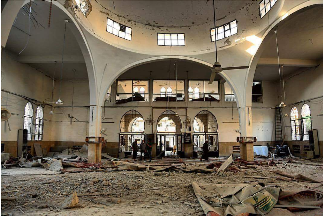
Interior damage to al-Rawda Mosque (Twitter ; July 21, 2016)
