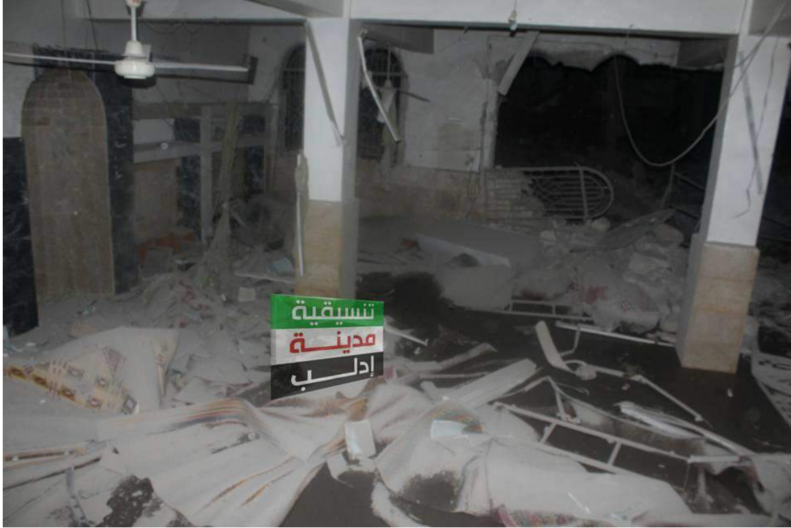
Damage to al-Hijazi Mosque (S.N.N; July 22, 2016)
