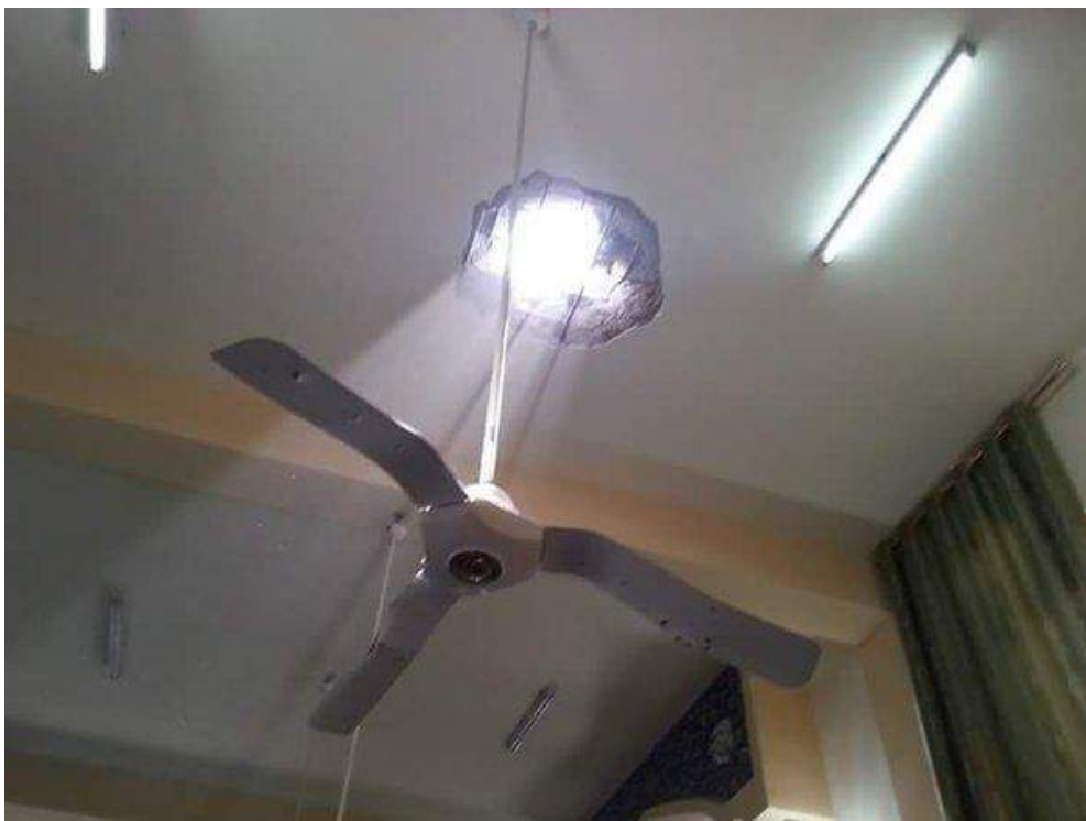
A photograph reporting to show a hole and damaged ceiling fan in Tawfiq Mosque (Twitter; August 14, 2015)
