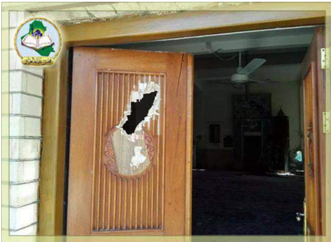
Damage to entrance of Sheikh Hamza Abbas al-Isawi Mosque (Majlis Iraq; August 17, 2014)
