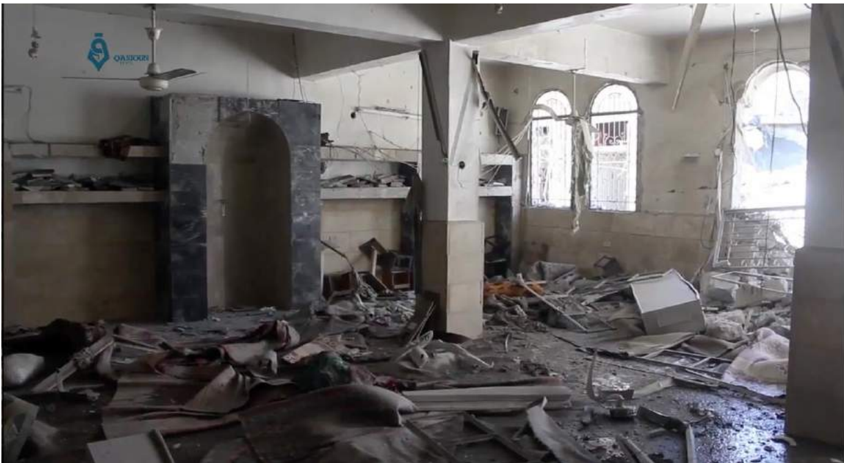
Video still of damage to al-Hijazi Mosque (Qasioun News Agency; July 22, 2016)
