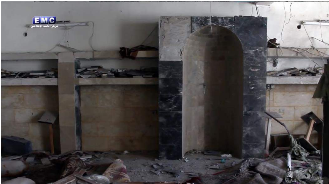
Video still of damage to the mihrab and interior of al-Hijazi Mosque (Edlib Media-Center; July 22, 2016)
