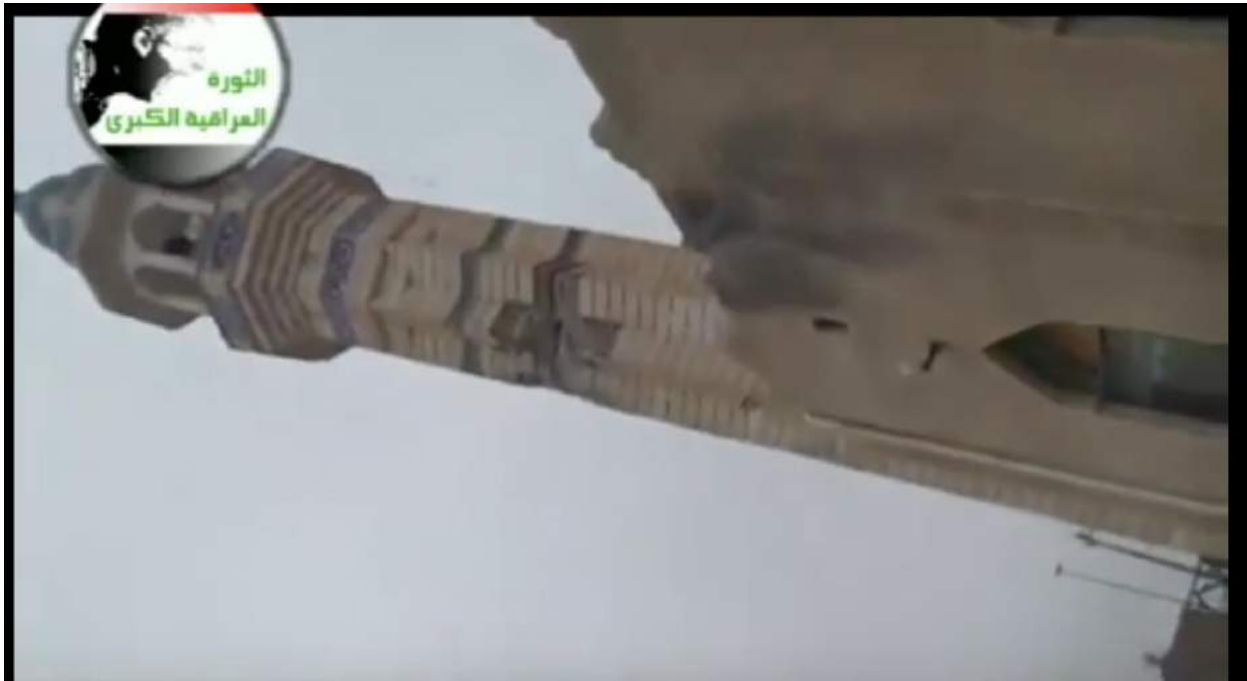
Damage to minaret and wall of Yusuf al-Sidiq Mosque (Thwar Aleashair/Youtube; January 6, 2014)
