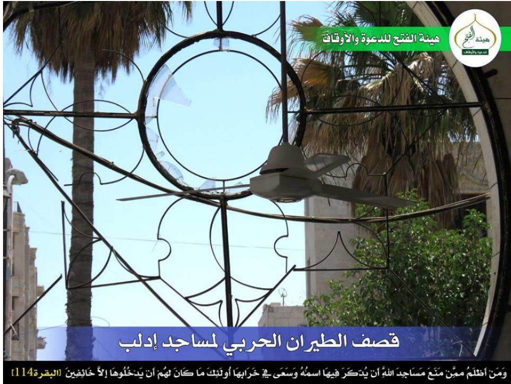
Previous damage to al-Rawda Mosque (Committee for Preaching and Endowment; June 7, 2016)
