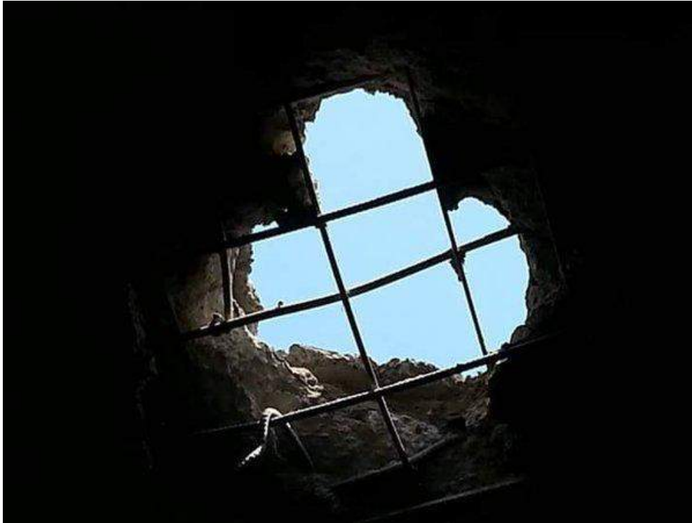
A photograph reporting to show a hole through the ceiling of Tawfiq Mosque (Twitter; August 14, 2015)
