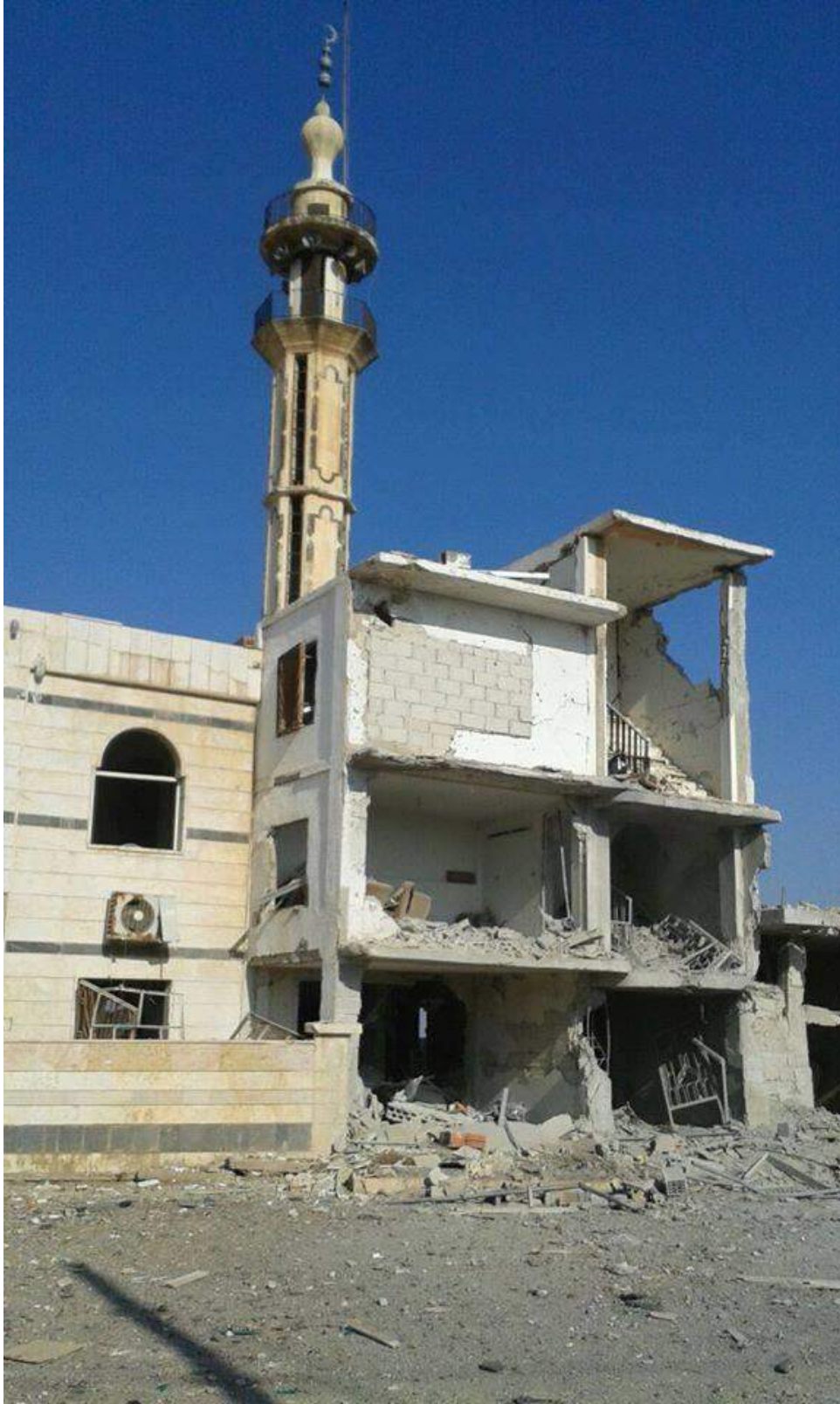
Damage to al-Musafir Mosque (SNHR; July 10, 2016)
