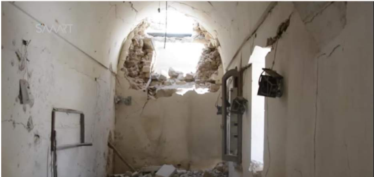
Video still of damage to al-Saleheen Mosque (SMART News Agency; July 16, 2016)
