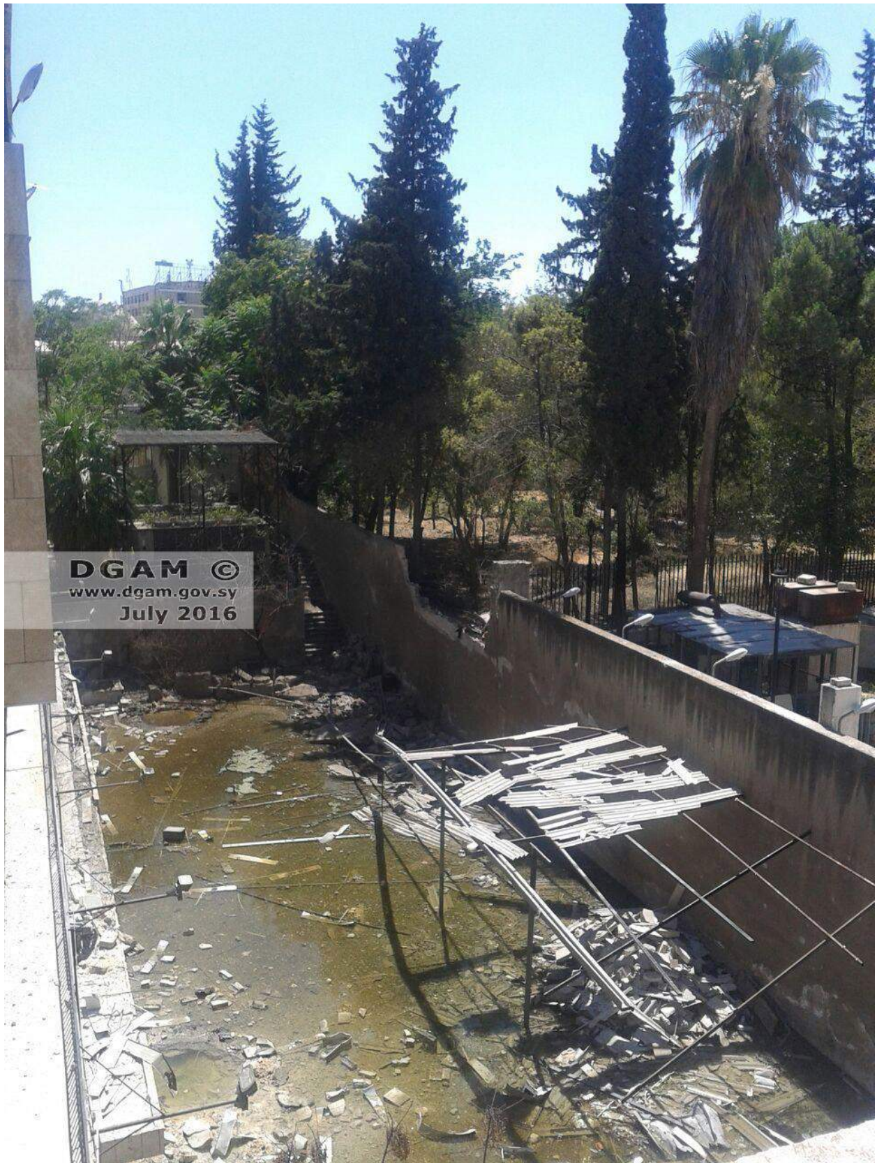
Damage to exterior of National Museum of Aleppo (DGAM; July 13, 2016)
