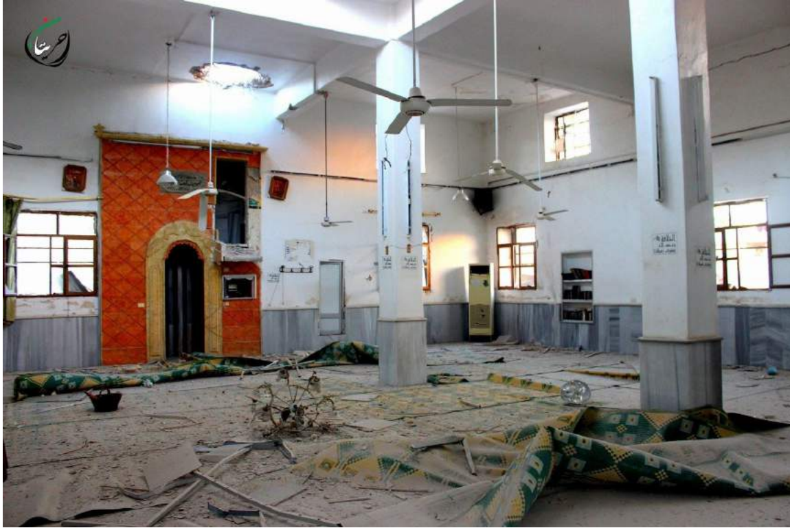
Damage to interior of Ali Sayyad Mosque in Hreitan (Hreitan City/Facebook; July 7, 2016)
