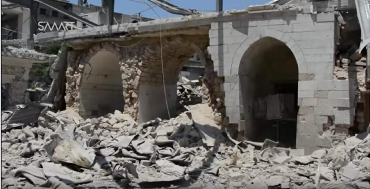
Video still of damage to exterior of al-Saleheen Mosque (SMART News Agency; July 16, 2016)
