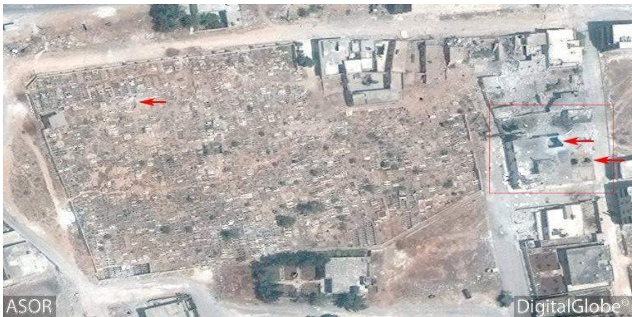
Ali Sayyad Mosque with additional damage especially to the eastern portion of the building. The red arrows point to the large hole in the roof, and the two small domes, which appear to have collapsed. There is also a new bomb crater in the cemetery (DigitalGlobe; July 7, 2016)
