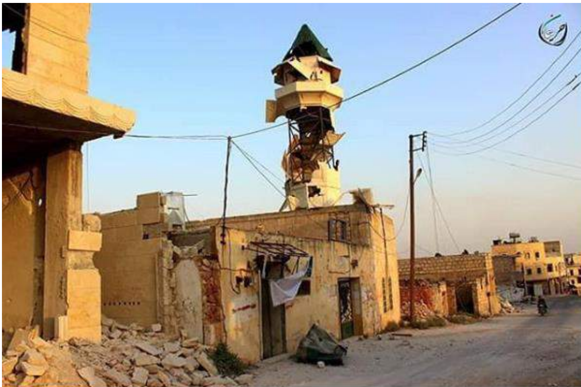
Damage to Khalid bin Waleed Mosque (Hraitan City; June 19, 2016)
