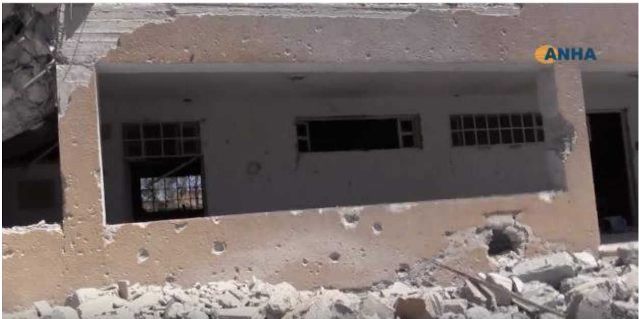
Severe damage to al-Sharaya School (ANHA; July 11, 2016)
