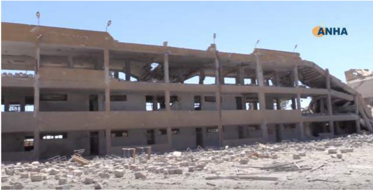
Severe damage to al-Sharaya School (ANHA; July 11, 2016)
