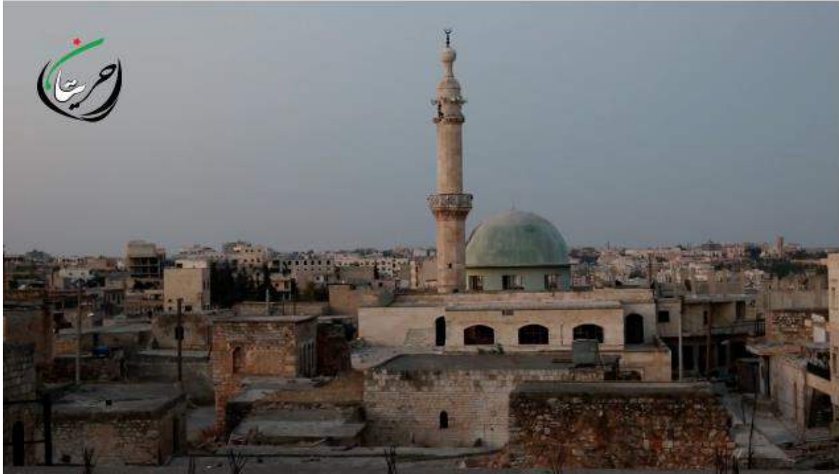
Video still of Abu Bakr al-Sedeiq Mosque showing light damage to the dome and minaret (Hreitan City; July 5, 2016)
