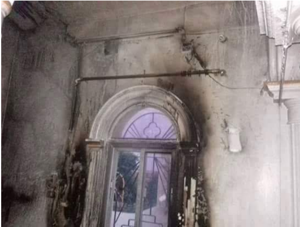
Fire and smoke damage in Mar Sharbel Church ( تراب ديريك الغالي /Facebook; July 18, 2016)
