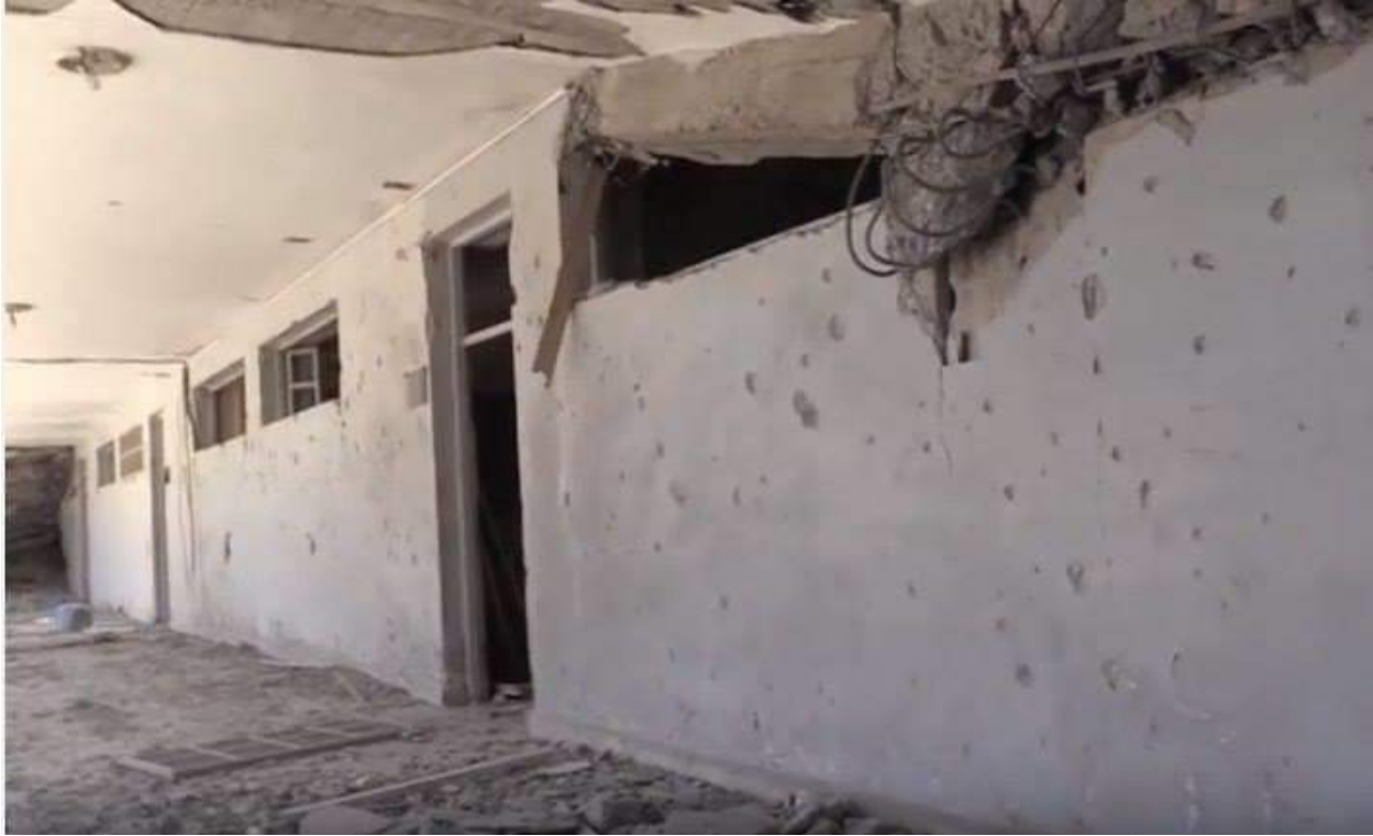
Severe damage to al-Sharaya School (Manbej Mubashar; July 13, 2016)
