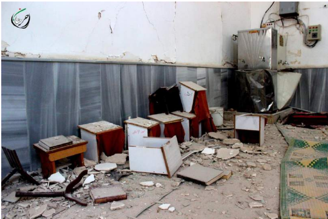
Damage to interior of Ali Sayyad Mosque in Hreitan (Hreitan City/Facebook; July 7, 2016)
