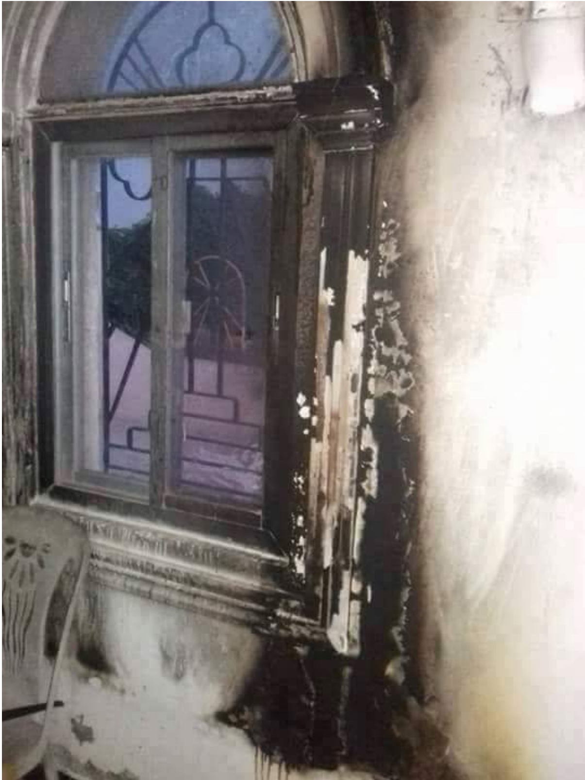
Fire damage to Mar Sharbel Church ( تراب ديريك الغالي /Facebook; July 18, 2016)
