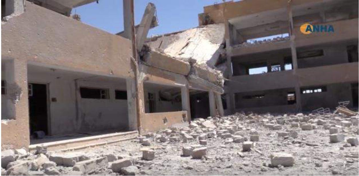
Severe damage to al-Sharaya School (ANHA; July 11, 2016)
