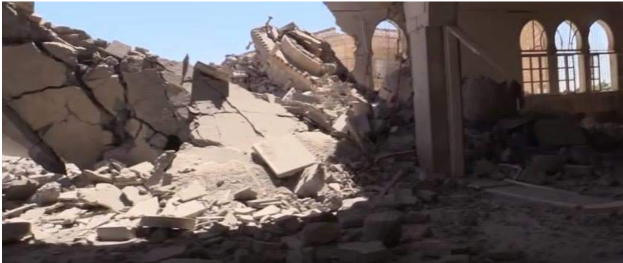
A collapsed wall at al-Miqdad Mosque (Manbej Mubashar; July 13, 2016)
