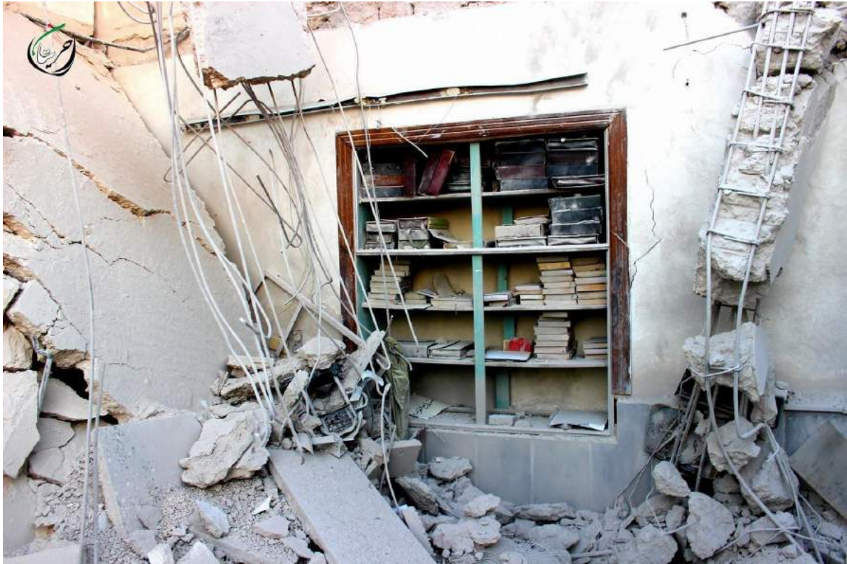
Severe damage to roof of Ali Sayyad Mosque in Hreitan (Hreitan City/Facebook; July 7, 2016)
