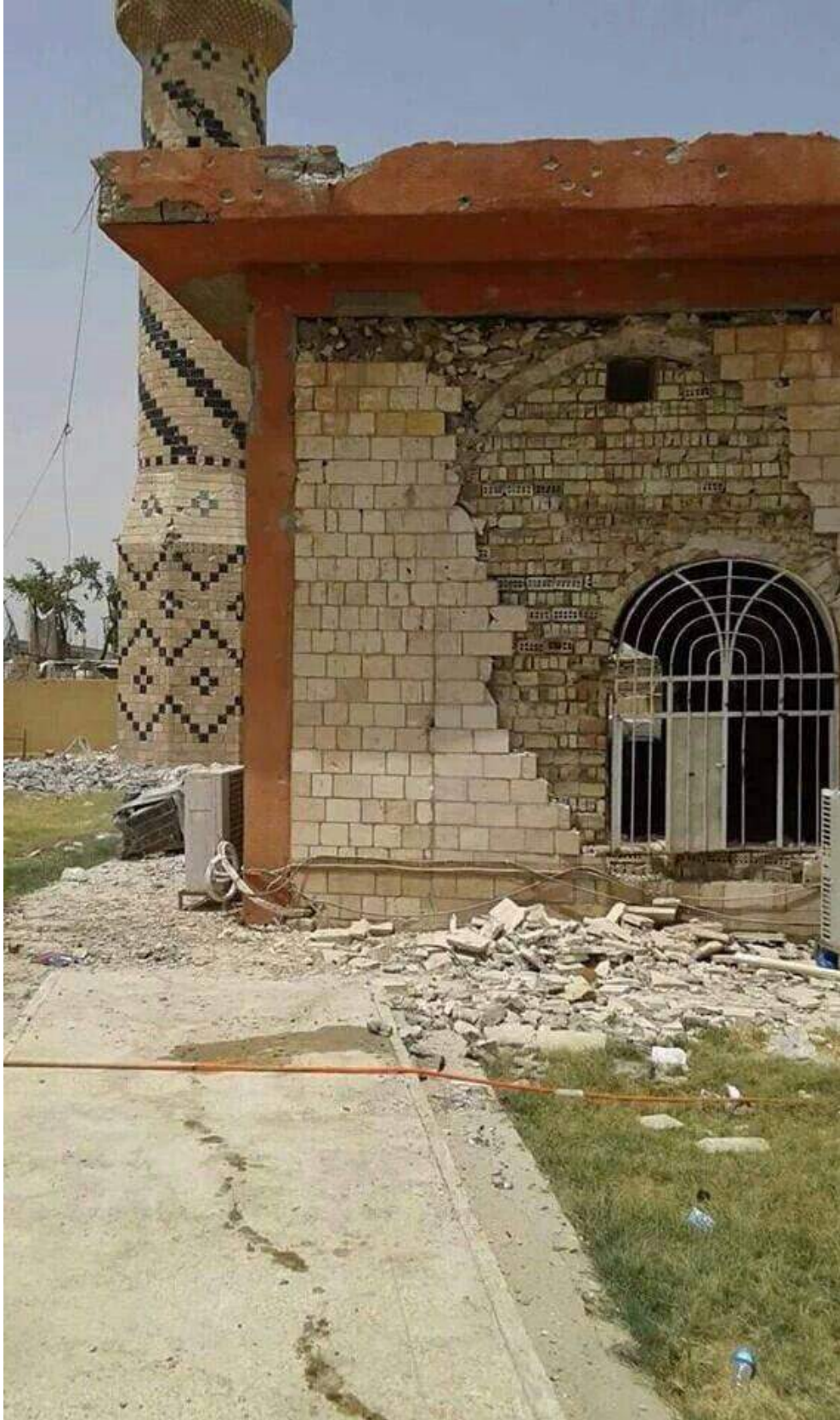
Damage to al-Fath al-Mudin Mosque (Twitter; July 10, 2016)
