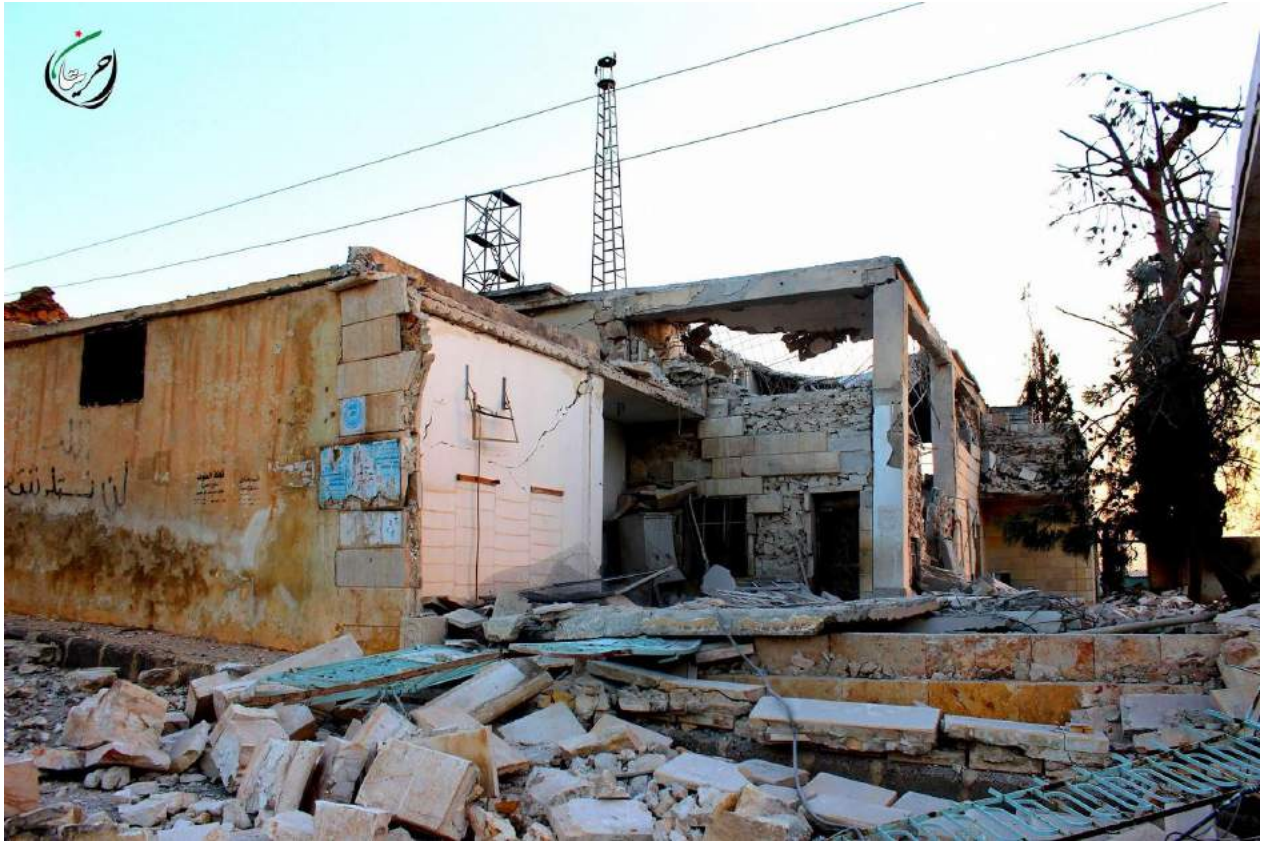
Severe damage to Ali Sayyad Mosque in Hreitan (Hreitan City/Facebook; July 7, 2016)
