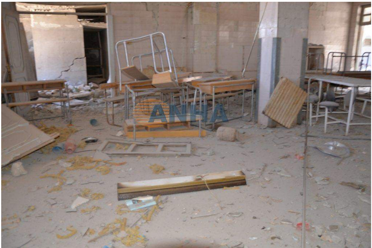
Severe damage to al-Sharaya School (Twitter; July 12, 2016)
