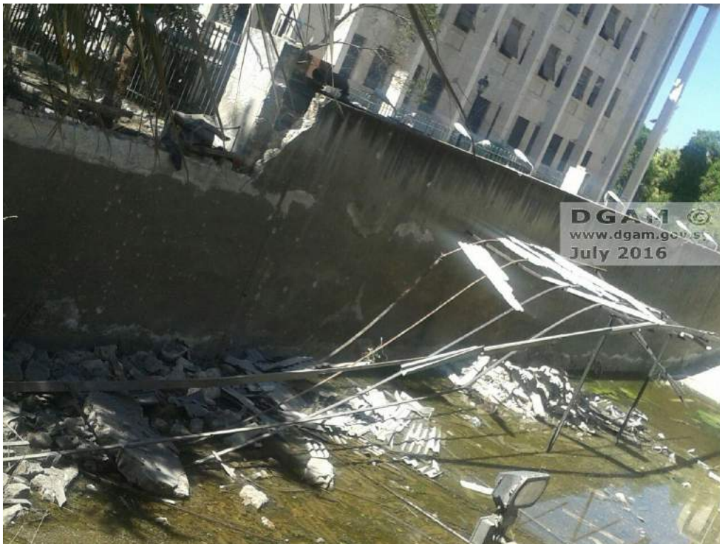
Damage to exterior of National Museum of Aleppo (DGAM; July 13, 2016)
