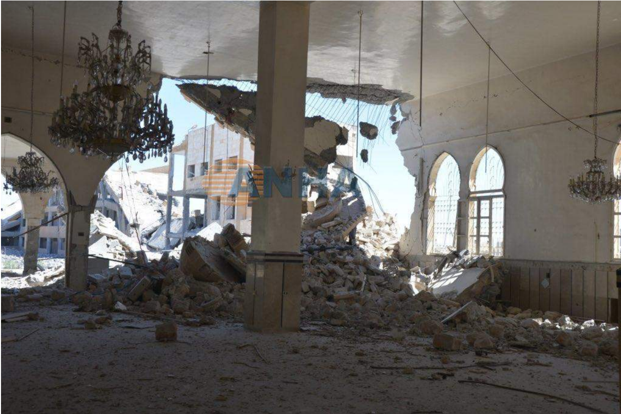
Detail of a collapsed wall at al-Miqdad Mosque (Twitter; July 12, 2016)
