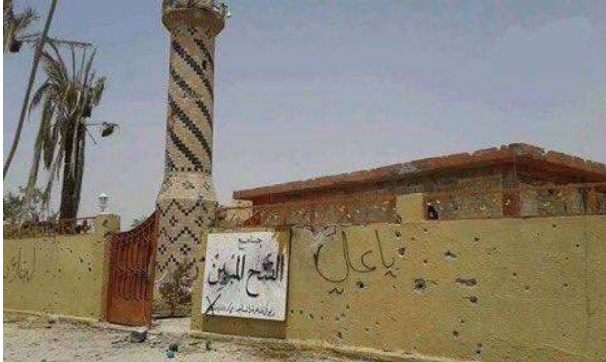
Gunfire damage and graffiti on exterior wall and minaret of al-Fath al-Mubin Mosque (Ahrar al-Rafidain Network for Human Rights/Facebook; July 4, 2016)
