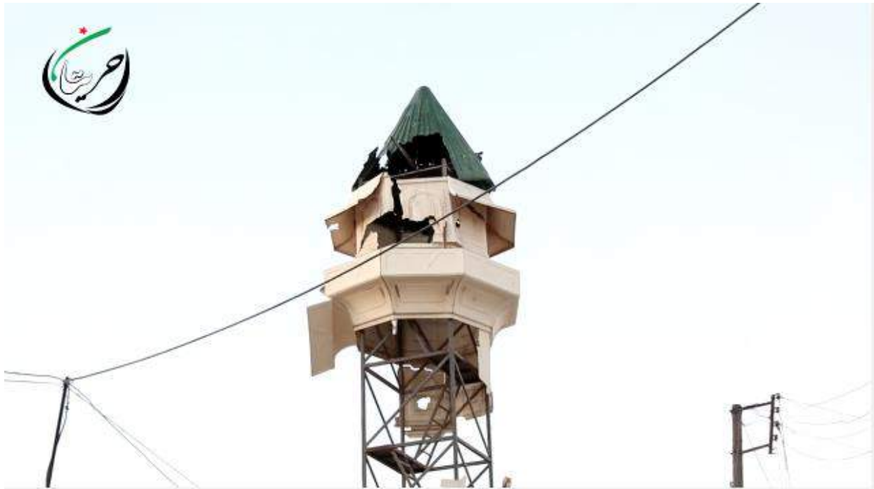
Video still of damage to Khalid bin Waleed Mosque (Hreitan City; July 5, 2016)
