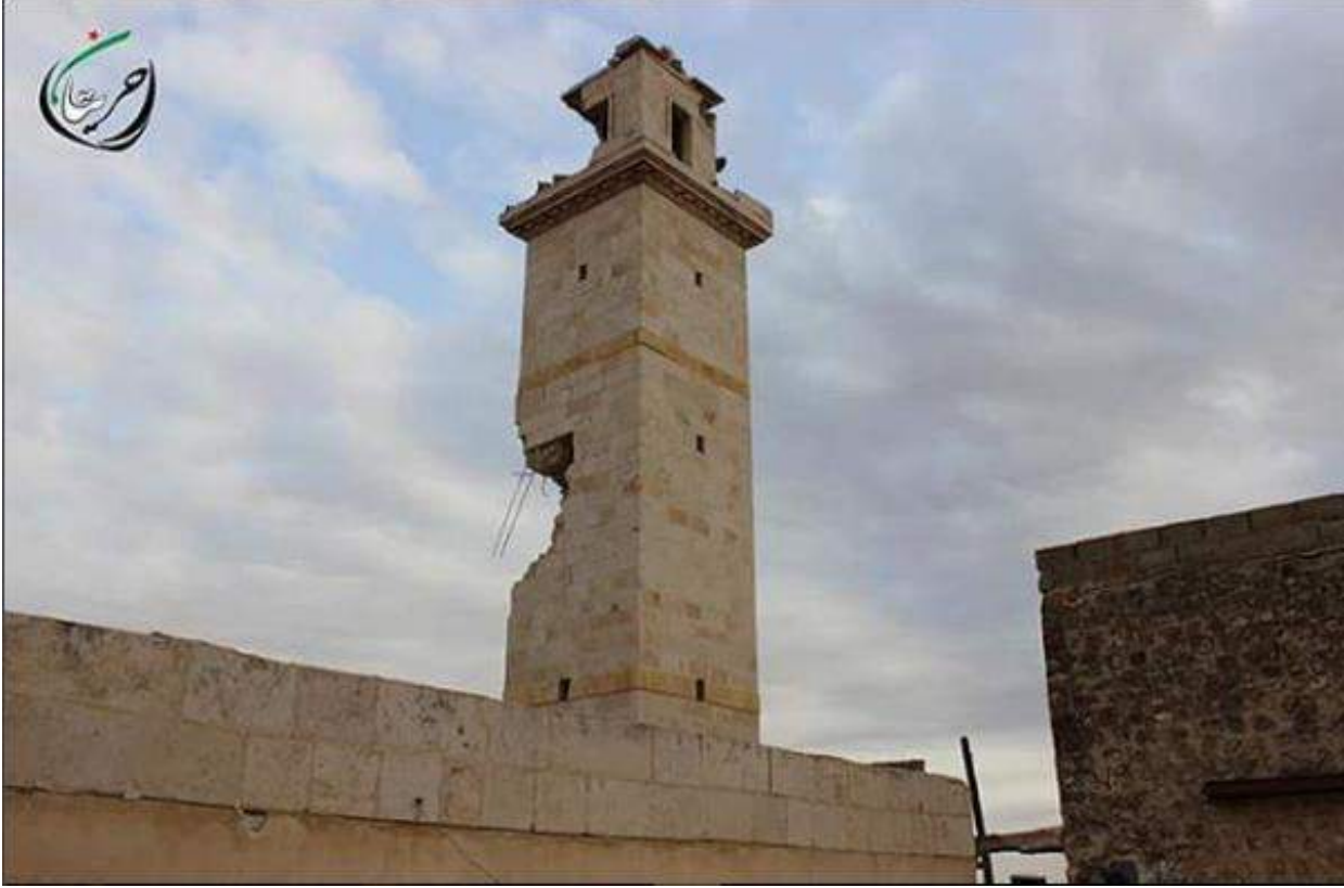
Damage to the minaret of the mosque in Tel Msebeen (Hreitan City; January 15, 2016)
