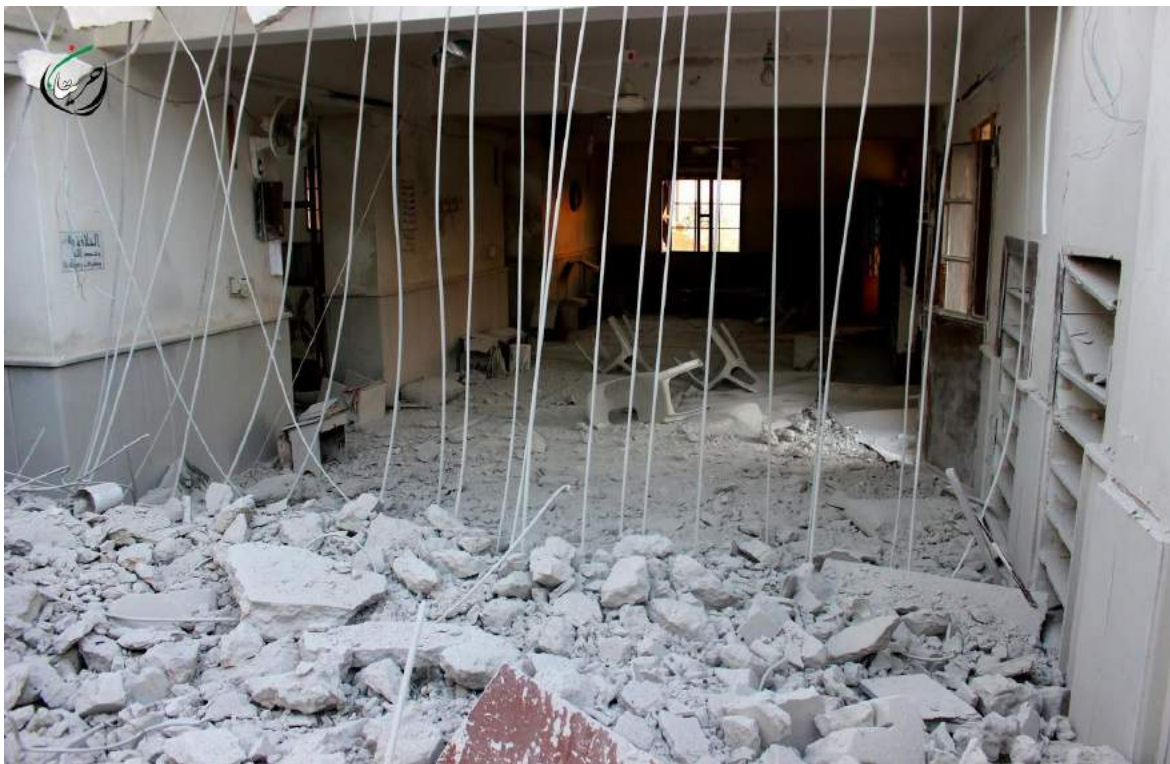
Severe damage to Ali Sayyad Mosque in Hreitan (Hreitan City/Facebook; July 7, 2016)
