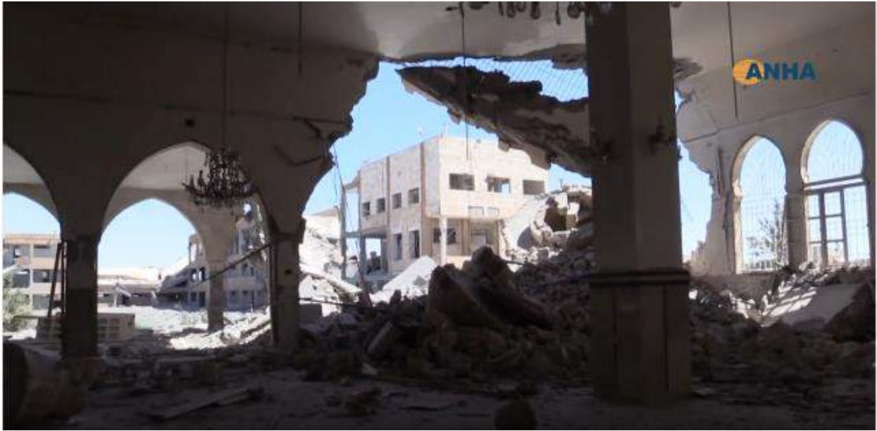
A collapsed wall at al-Miqdad Mosque (ANHA; July 11, 2016)
