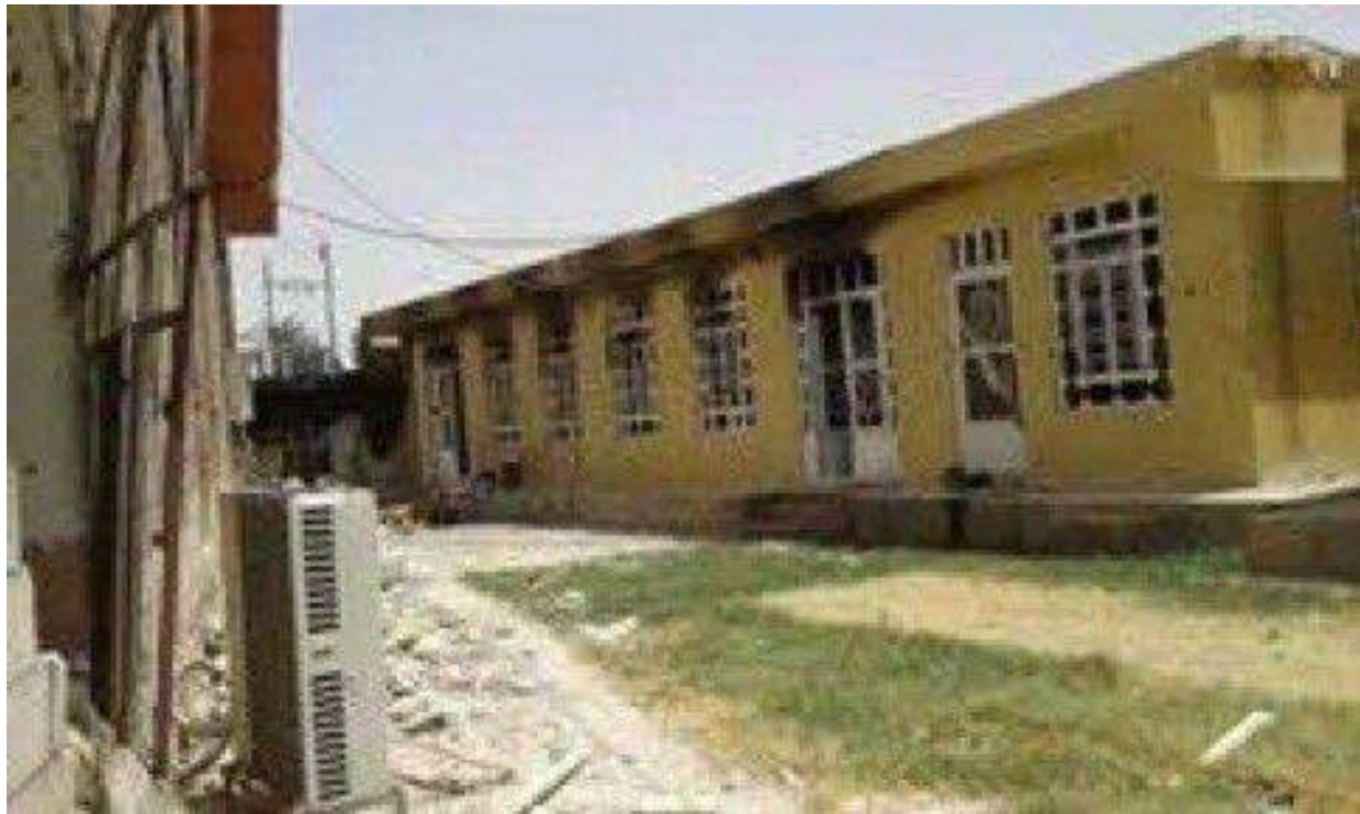
Fire damage to part of al-Fath al-Mubin Mosque complex (Ahrar al-Rafidain Network for Human Rights/Facebook; July 4, 2016)
