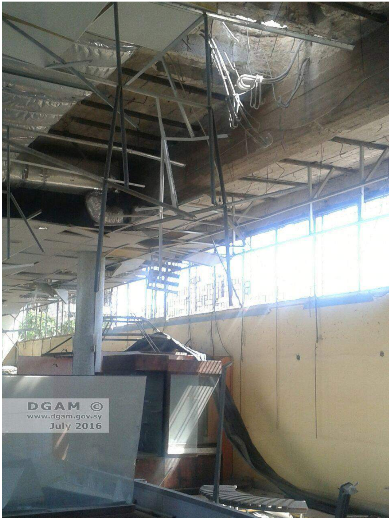
Damage to interior of National Museum of Aleppo (DGAM; July 13, 2016)
