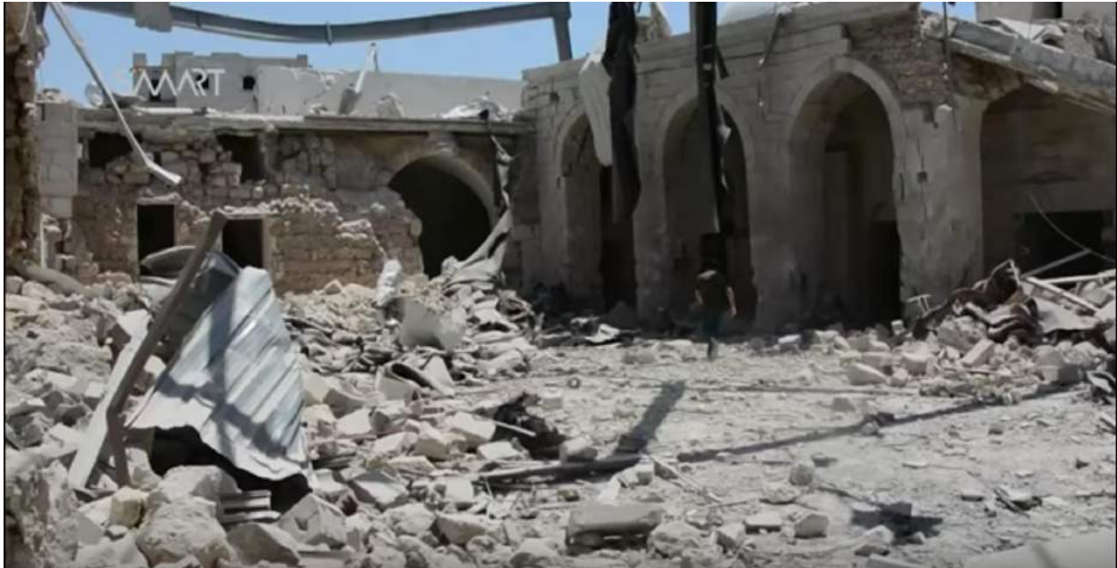
Video still of damage to exterior of al-Saleheen Mosque (SMART News Agency; July 16, 2016)
