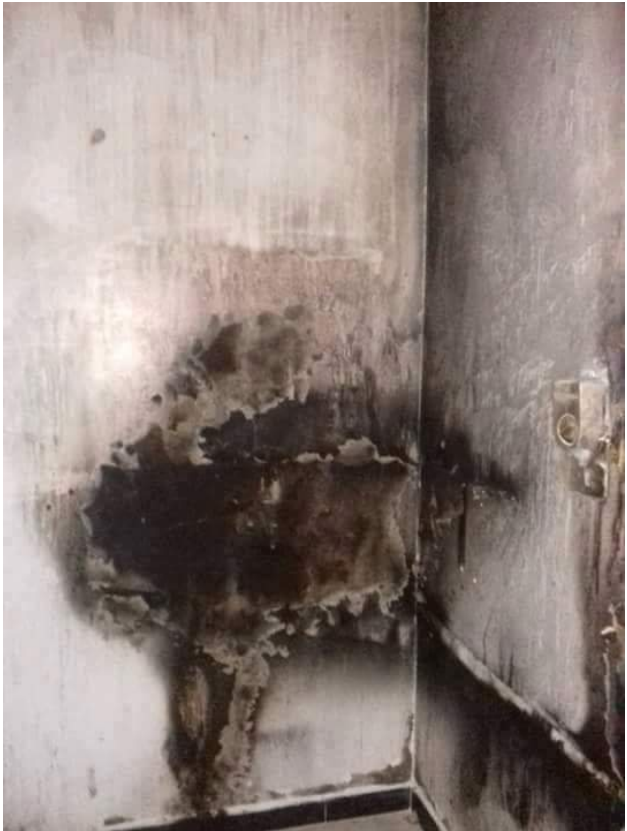
Fire damage in Mar Sharbel Church ( تراب ديريك الغالي /Facebook; July 18, 2016)
