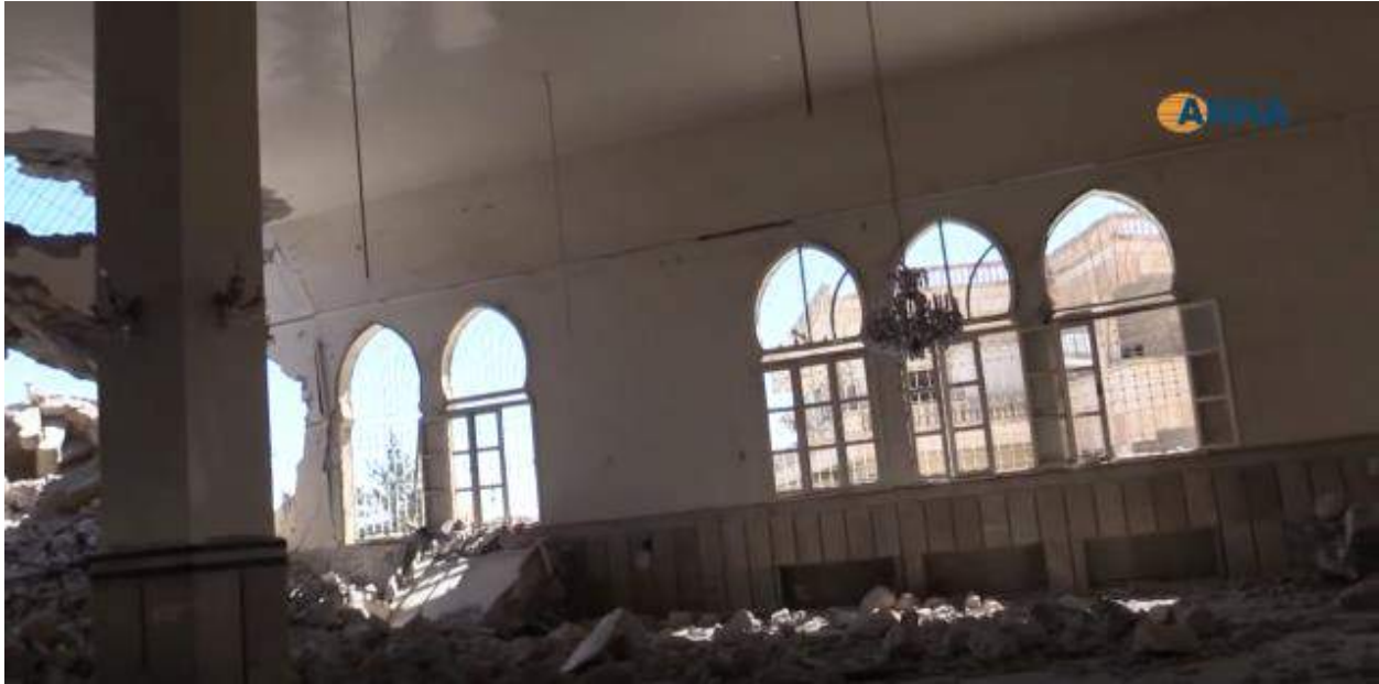
Damage to al-Miqdad Mosque (ANHA; July 11, 2016)
