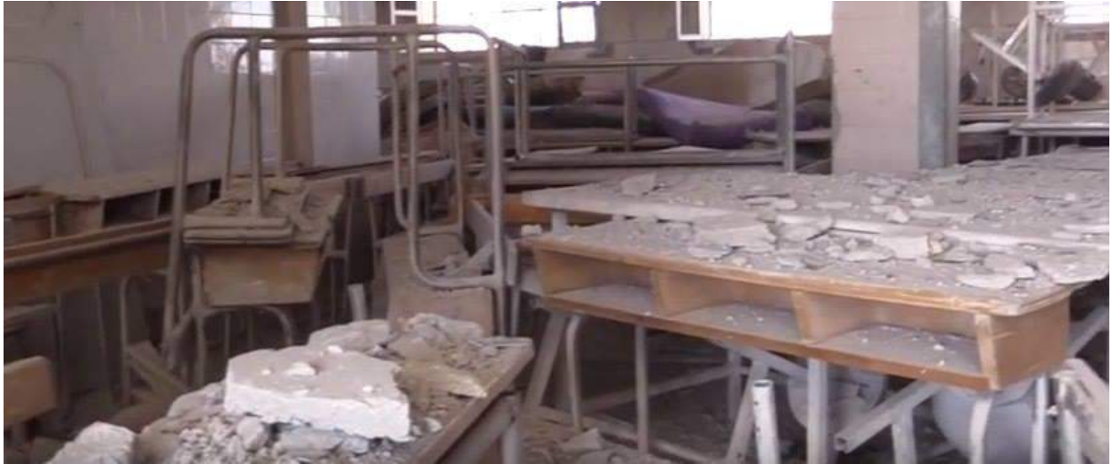
Severe damage to al-Sharaya School (Manbej Mubashar; July 13, 2016)
