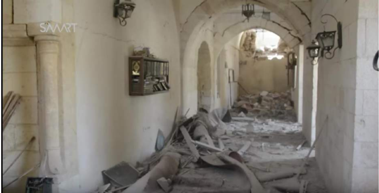
Video still of damage to al-Saleheen Mosque (SMART News Agency; July 16, 2016)
