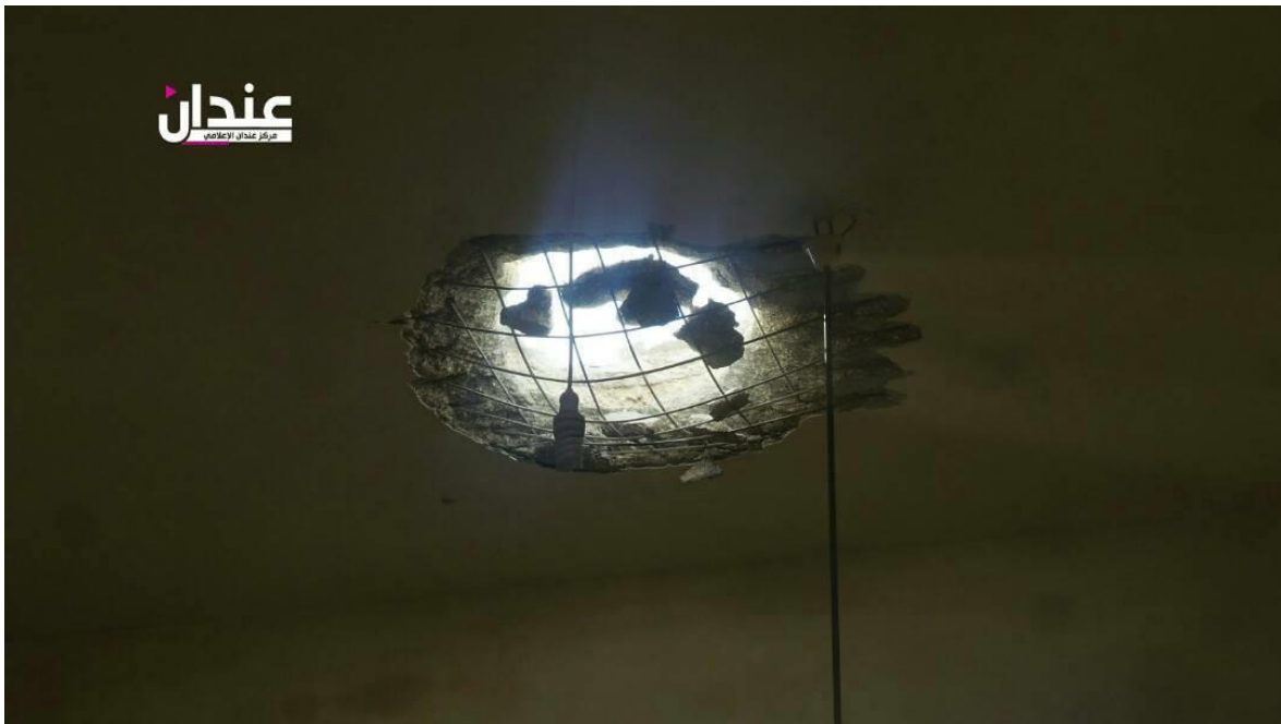
Damage to mosque ceiling (Anadan Media Center; October 12, 2017)
