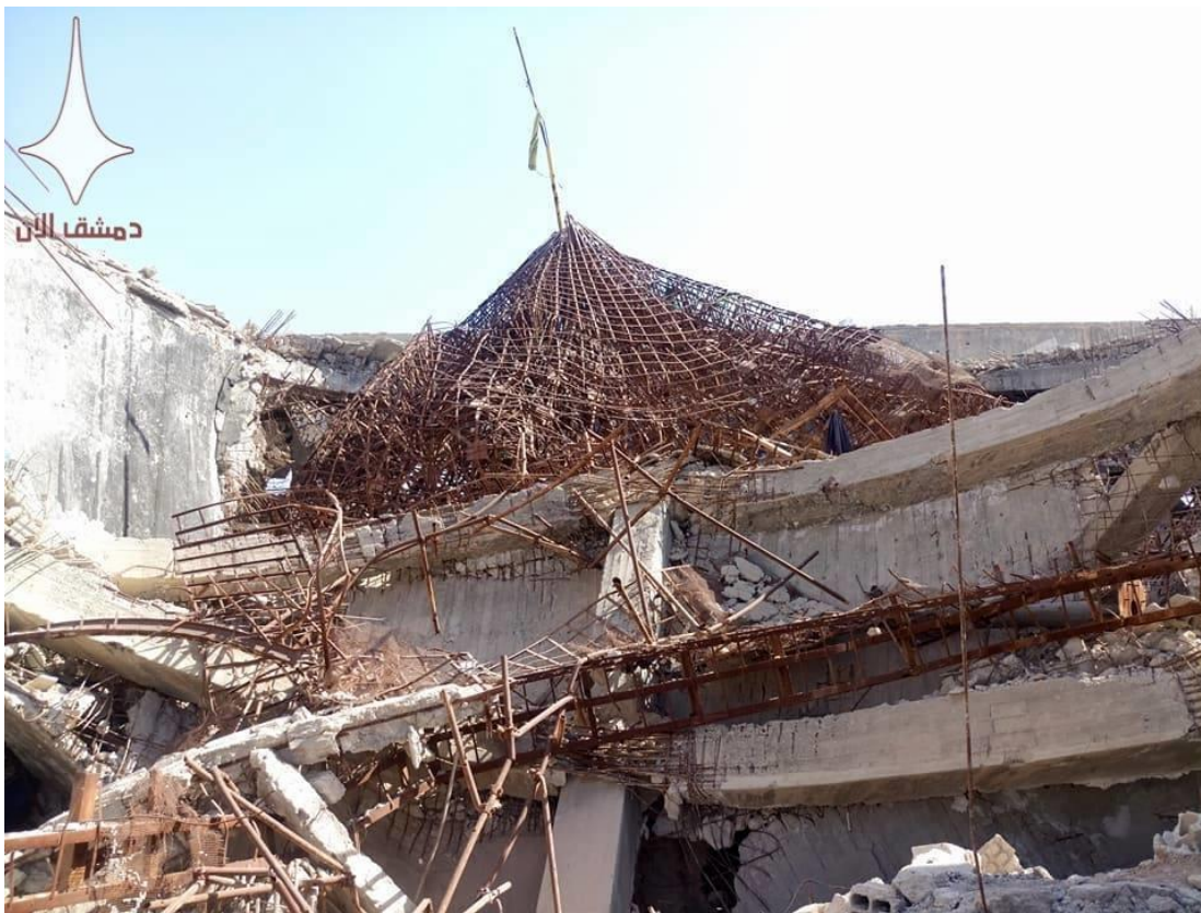
Photograph of damage to the shrine, with remnants of the destroyed dome in foreground (Private Facebook Account; October 8, 2017)
