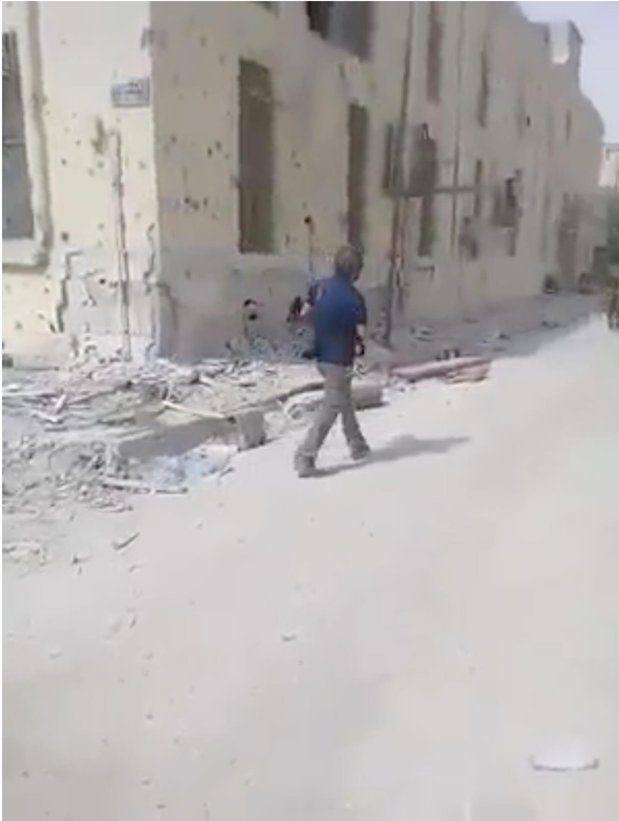
Video still of damage from small-arms fire, seen from the southeast (RBSS; October 4, 2017)
