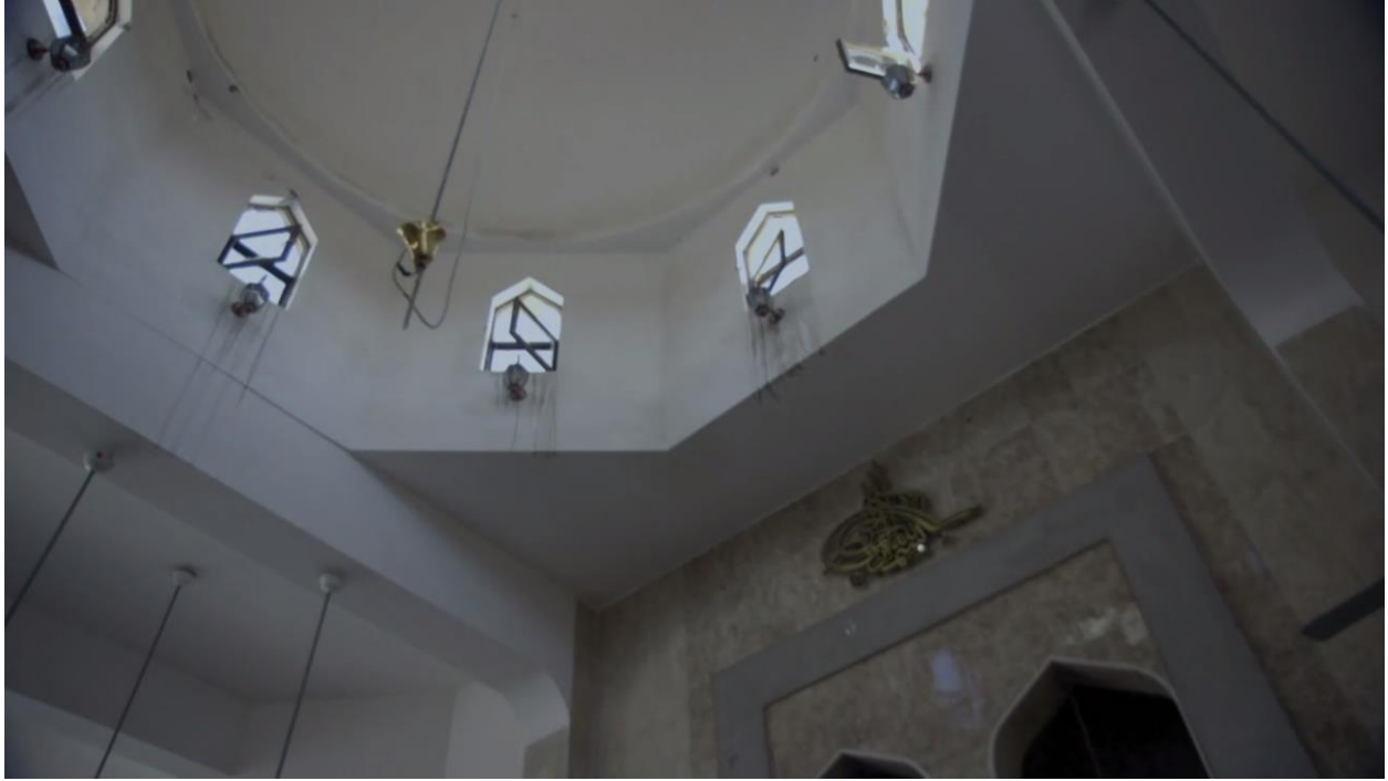
Video still of the mosque's interior. Note the water damage near the open windows (VICE News; October 13, 2017)
