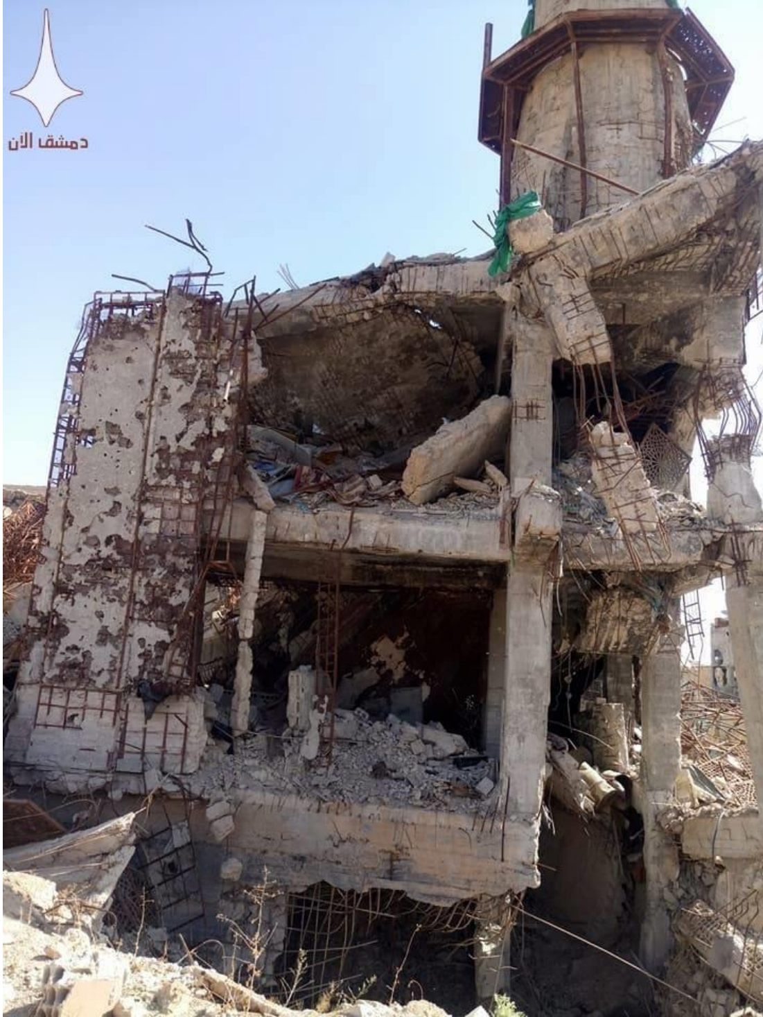
Photograph of damage to the shrine's minaret (Private Facebook Account; October 8, 2017)
