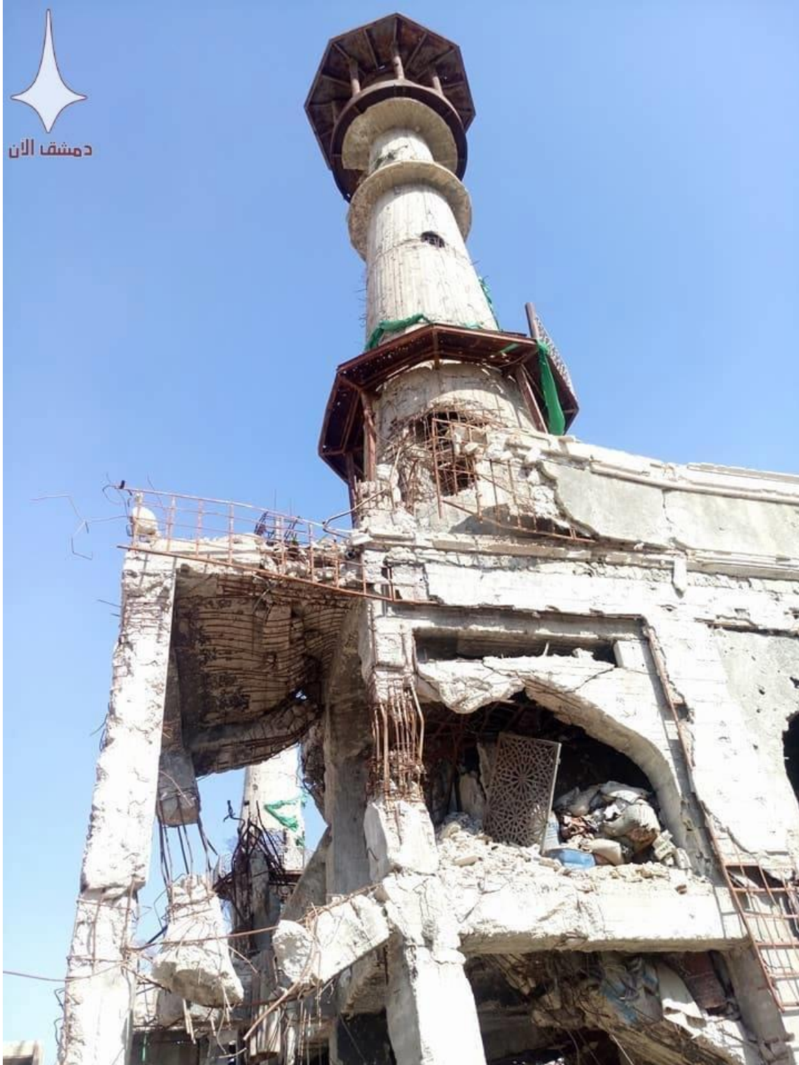
Photograph of damage to the shrine below the minaret (Private Facebook Account; October 8, 2017)
