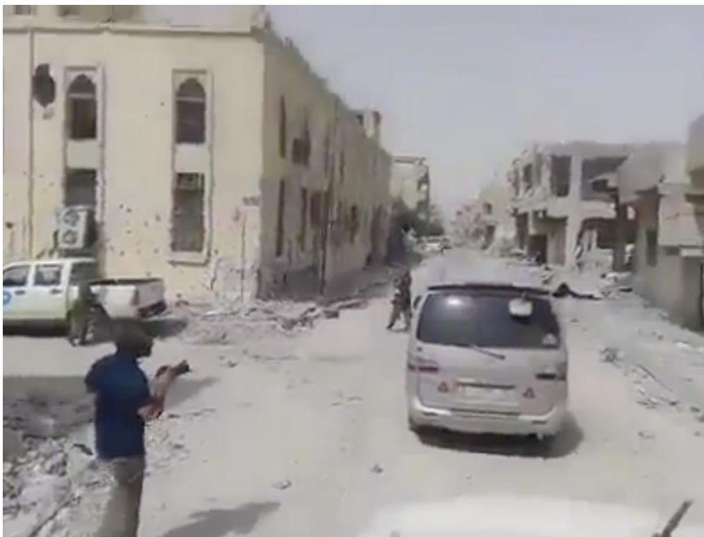
Video still of damage from small-arms fire, seen from the south. Note the larger hole near the second story window (RBSS; October 4, 2017)
