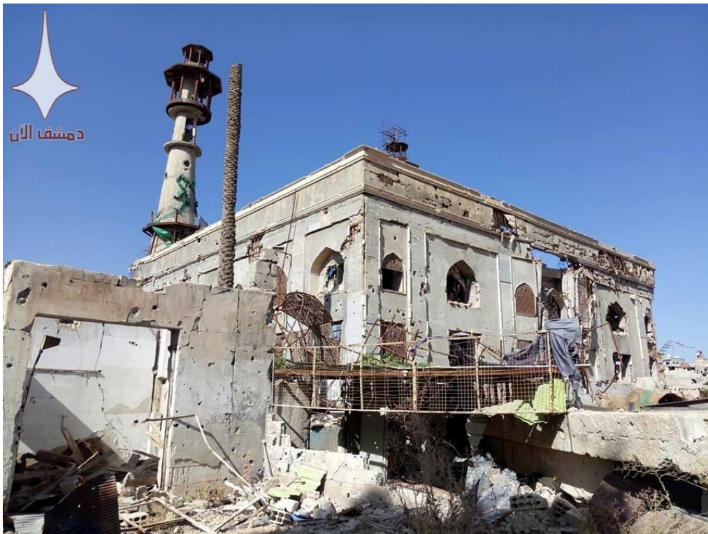
Photograph of damage to the shrine, seen from rear of the structure (Private Facebook Account; October 8, 2017)
