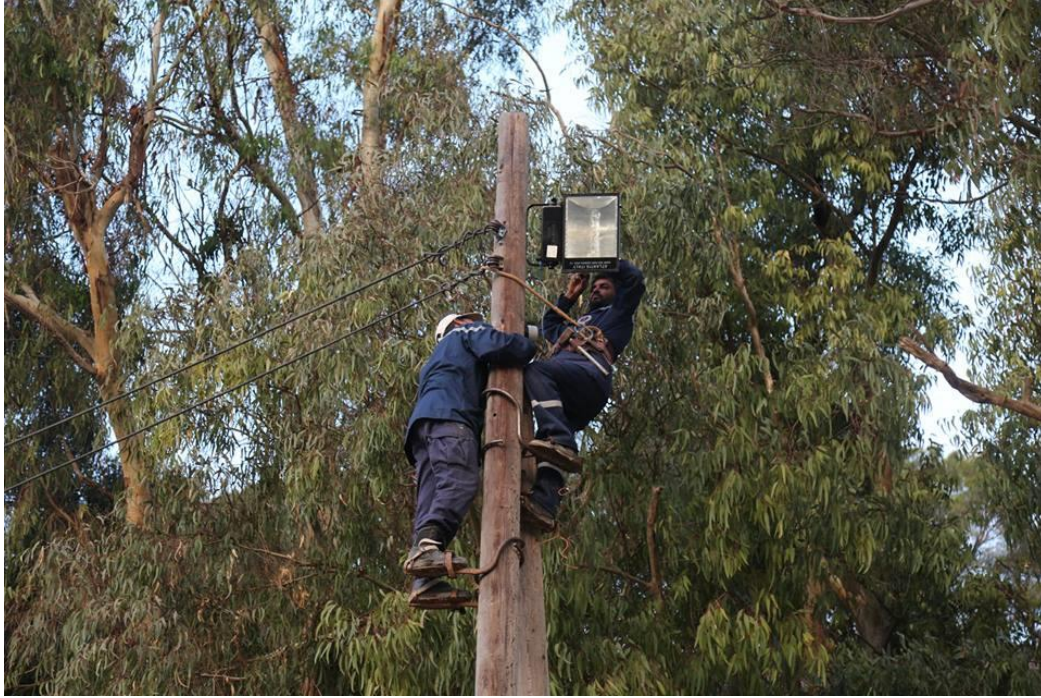
Crew installs new lights adjacent to the Sanctuary of Apollo (DoA Shahat; October. 5, 2017)
