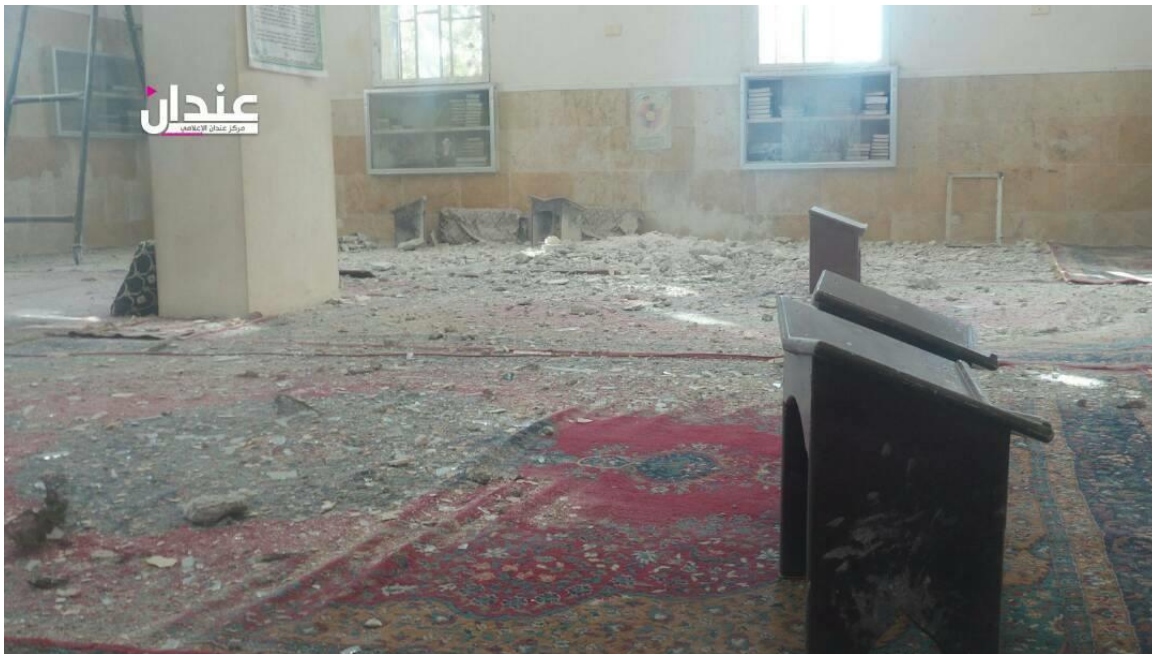
Damage to the interior of Abu Bakr al-Siddiq Mosque (Anadan Media Center; October 11, 2017)
