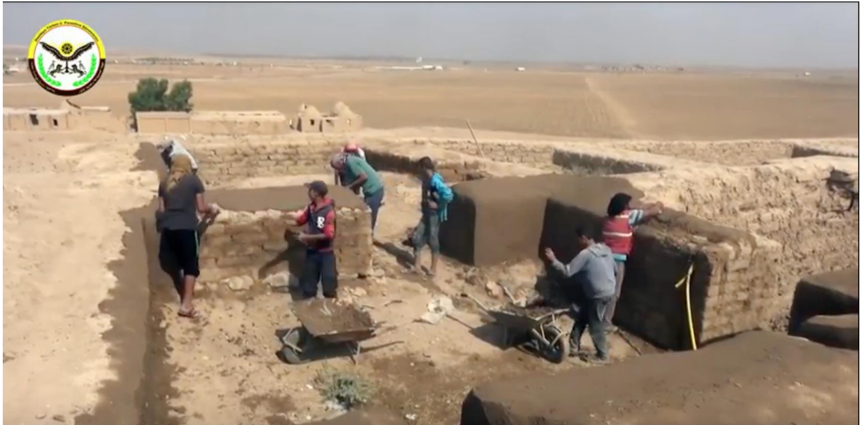
Video still of restoration work on mudbrick walls at Tell Beydar (ATPA/Youtube; October 2, 2017)
