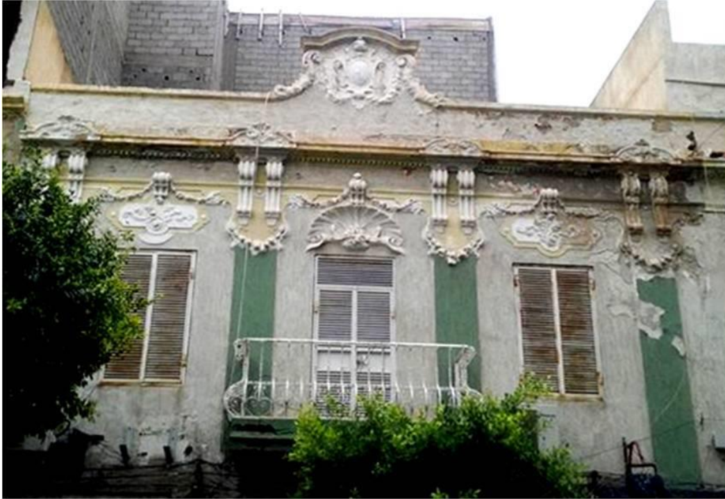
Historic building from the Italian period with new construction behind (Private Facebook Account; October. 3, 2017)
