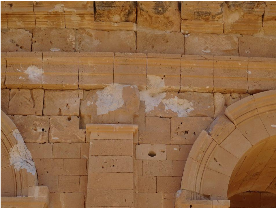
Detail of damage to the Sabratha theater (Hafed Walda; October 9, 2017)
