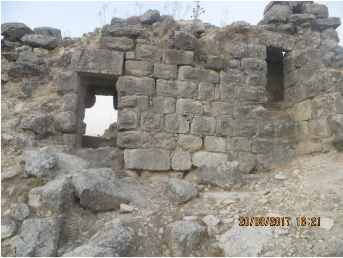
Damage due to weathering effects
