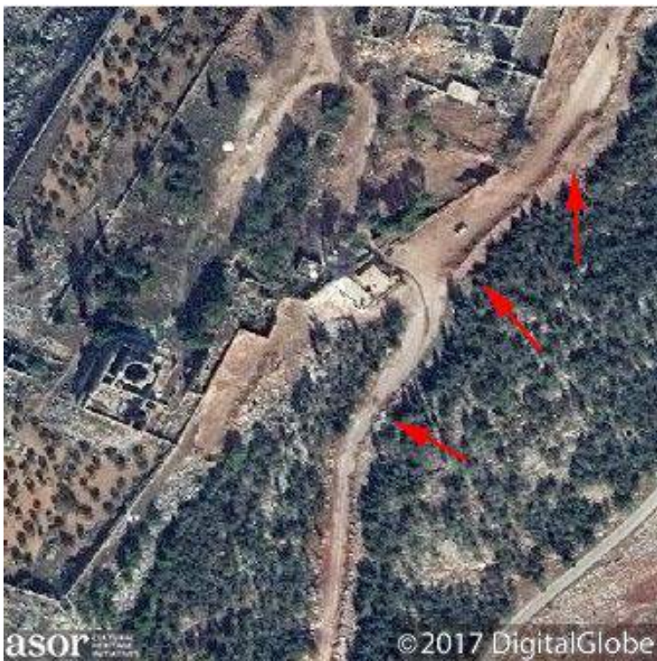
Area east of site after road construction and earthworks building has begun (DigitalGlobe NextView License; November 9, 2017)
