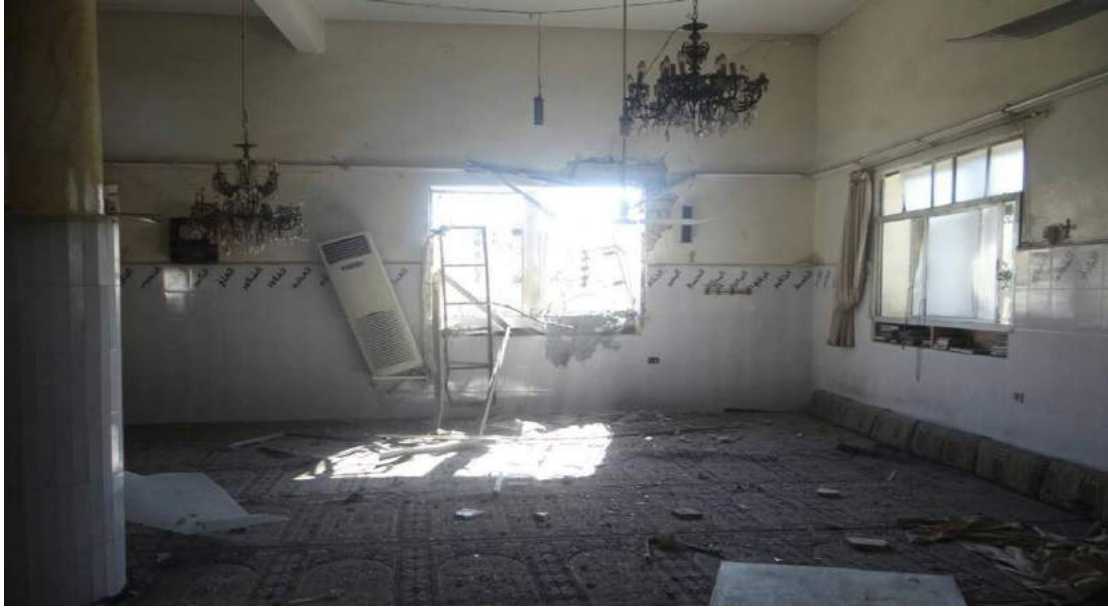
A view of the damaged window and associated debris, seen from the north (SNHR; November 11, 2017)
