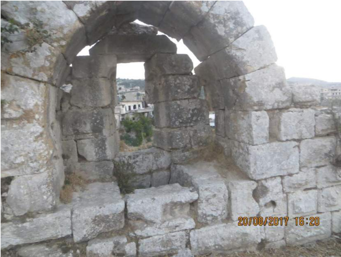
Collapse due to natural causes
