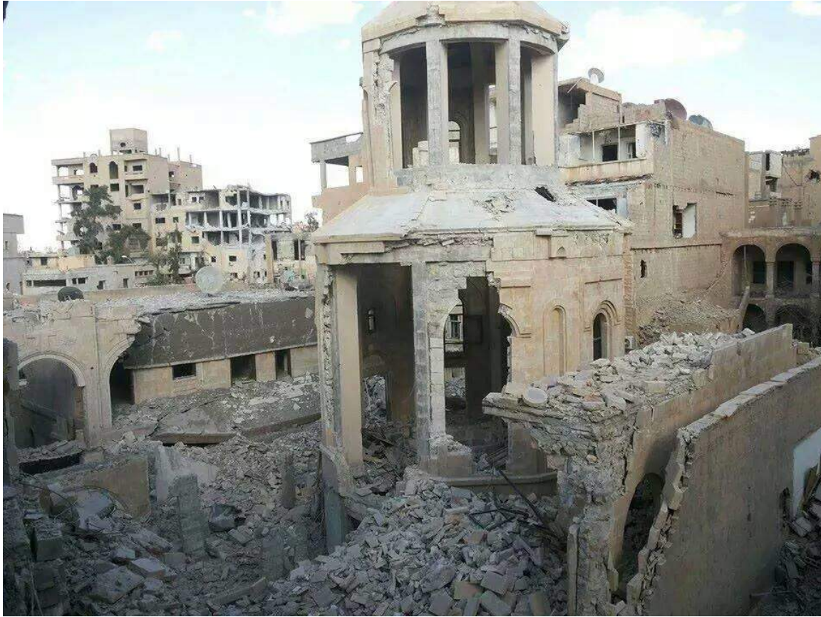
One of the first photographs of damage to the exterior of the church (Armenian Weekly/Al-Masdar; September 24, 2014)
