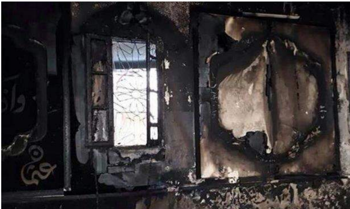
Fire damage to the interior of the mosque (Al Wasat; November 28, 2017)
