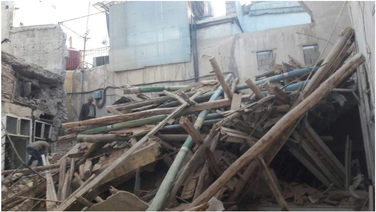
Collapse of house in Old Damascus (DGAM; November 2, 2017)
