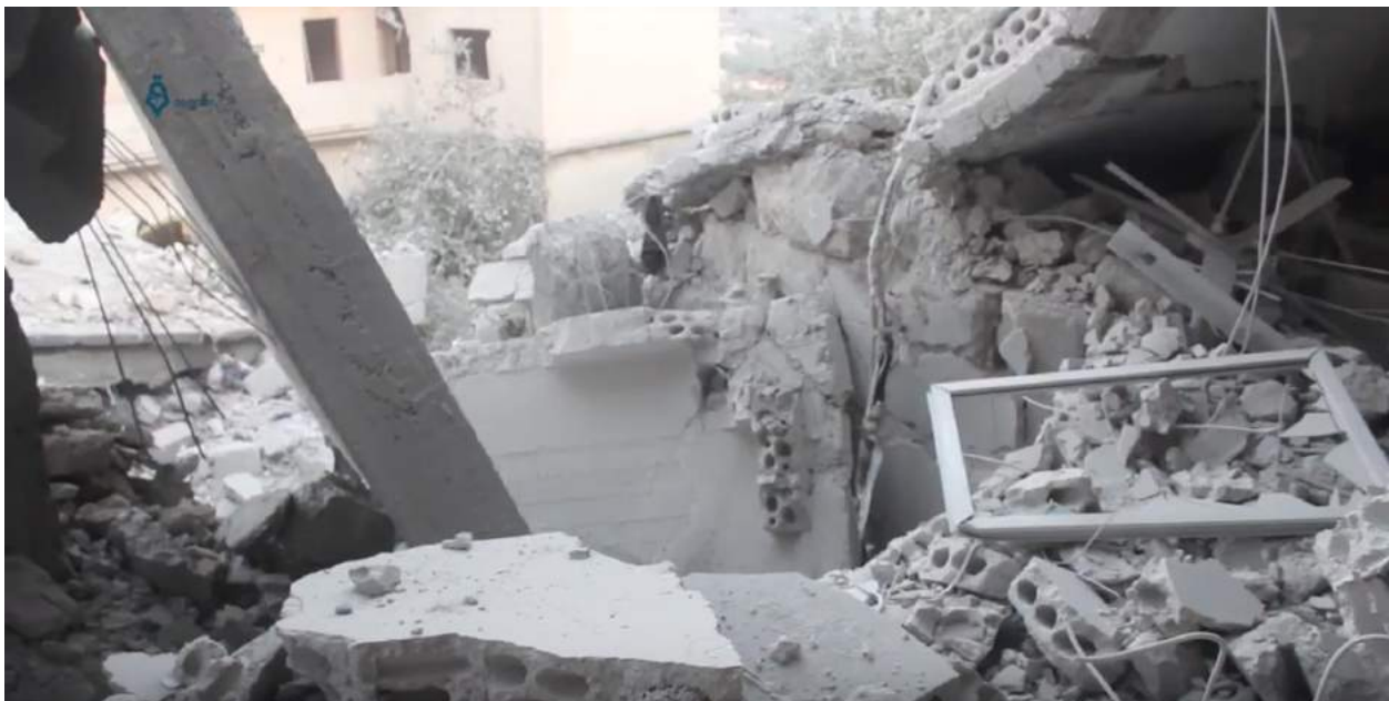
Video still of damage to the exterior of al-Kabir Mosque (Qasioun News Agency; September 29, 2017)
