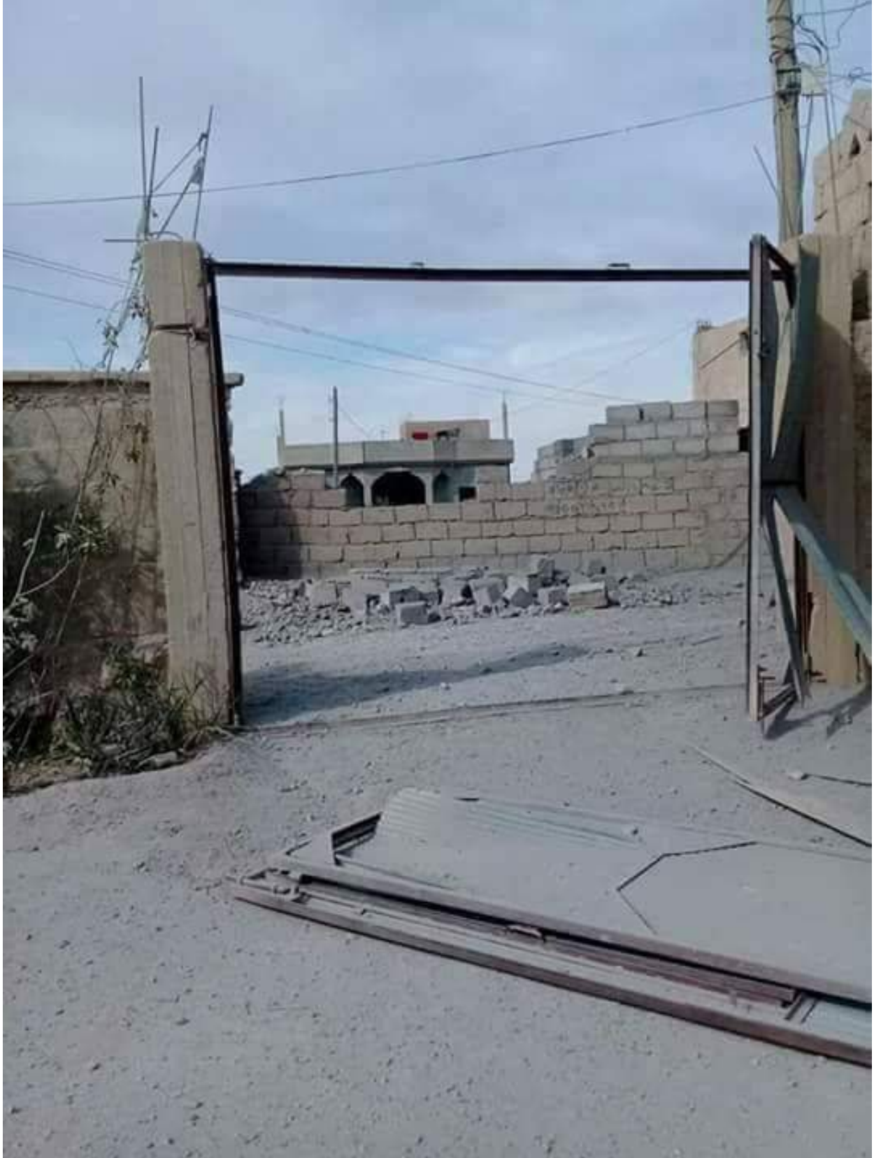
Damage to entrance gate of al-Taas Mosque (Euphrates Post; November 1, 2017)
