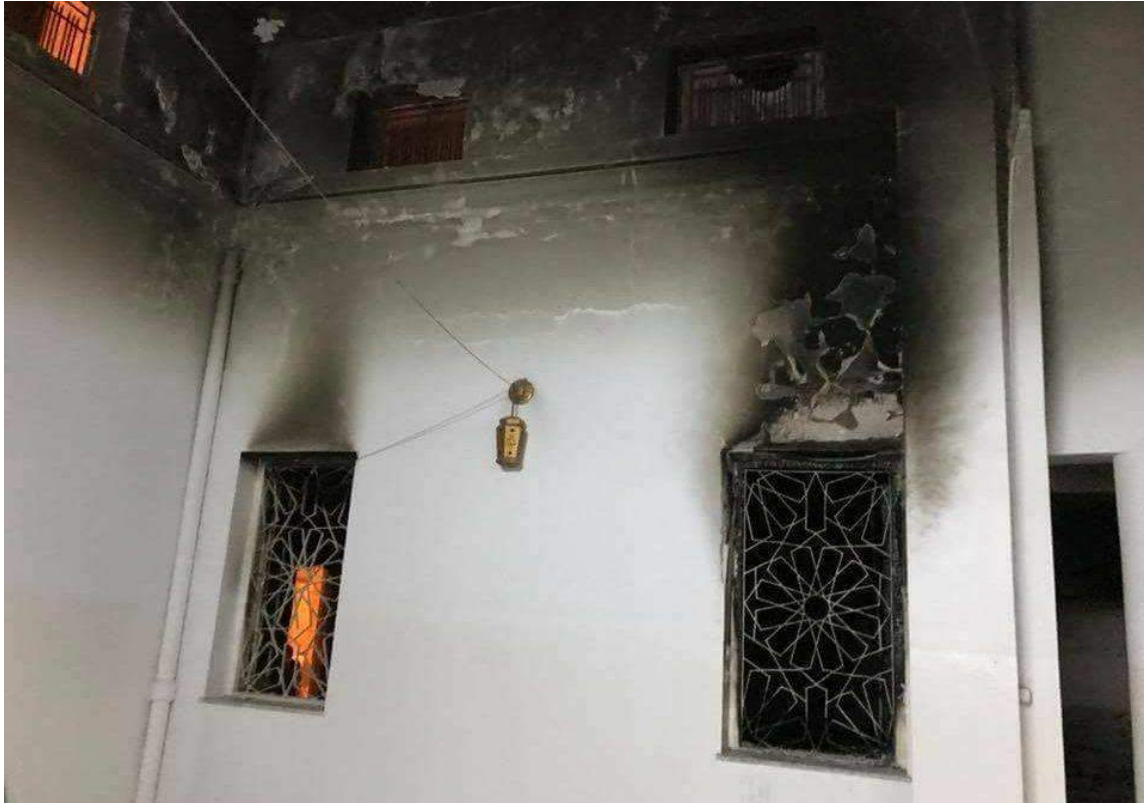
Fire damage on exterior of al-Sheikha Radiya Mosque (Qana' Libya; November 28, 2017)
