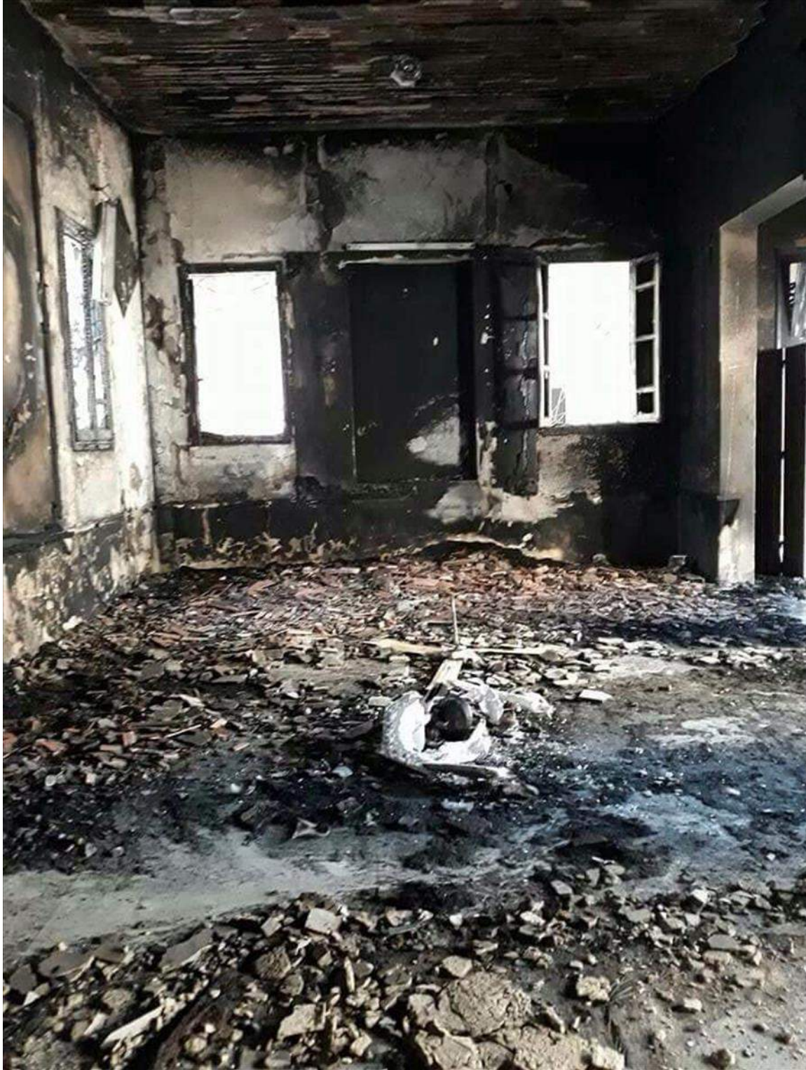
Fire damage to the interior of the mosque (Al Wasat, November 28, 2017)
