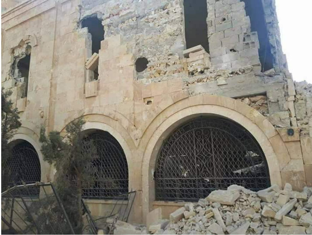
Damage to the exterior of the church (Armenian Weekly/Al-Masdar; November 6, 2017)
