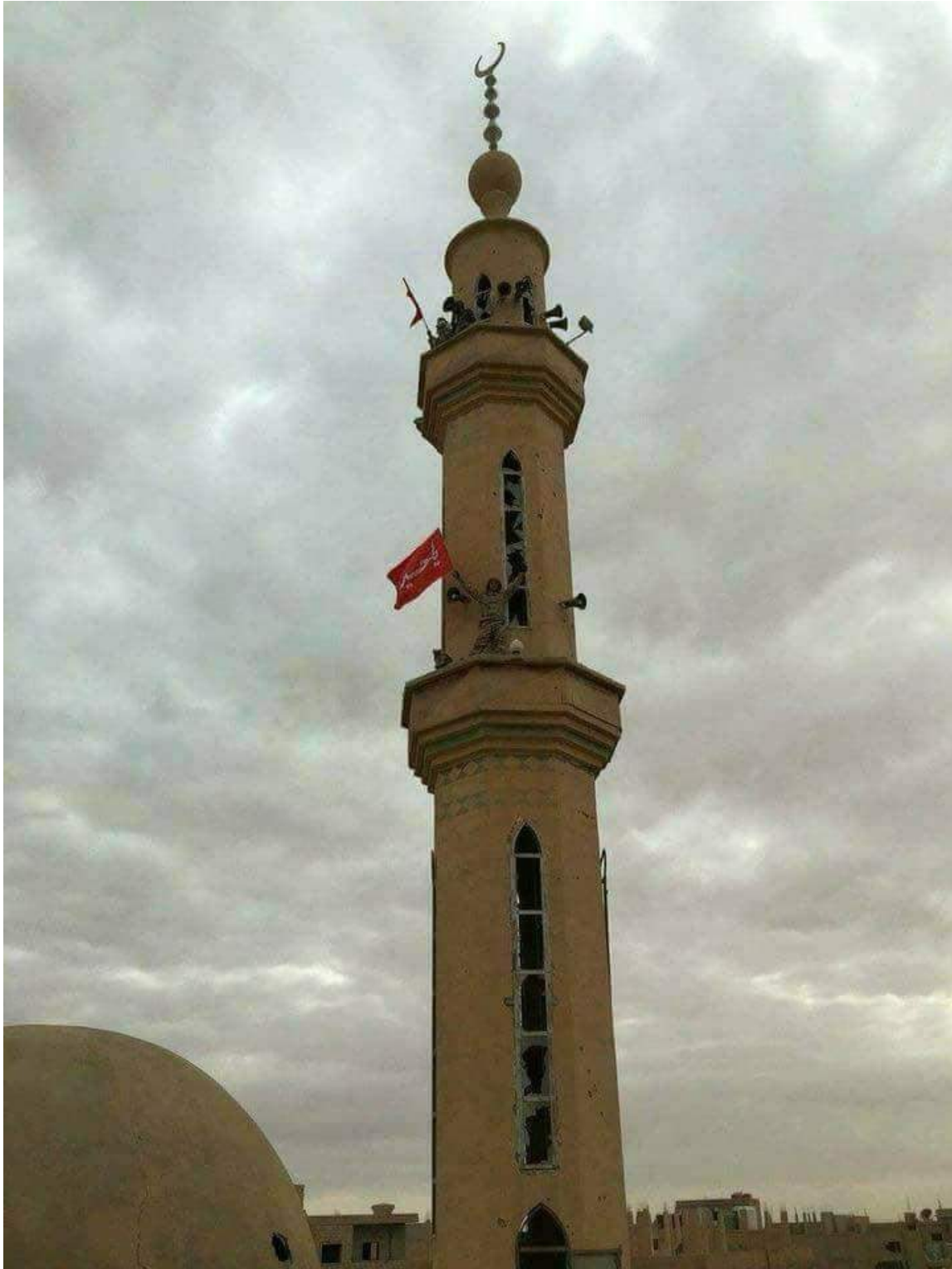
Damage seen to the minaret (al-Bukamal al-Mayadin al-Balad; November 28, 2017)
