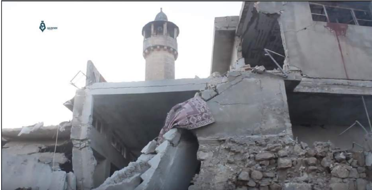
Video still of damage to the exterior of al-Kabir Mosque (Qasioun News Agency; September 29, 2017)
