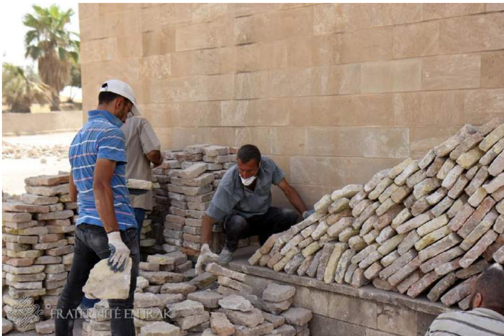
Workers sort bricks for use during reconstruction of Mar Behnam Monastery (Fraternité in Irak; October 27, 2017)
