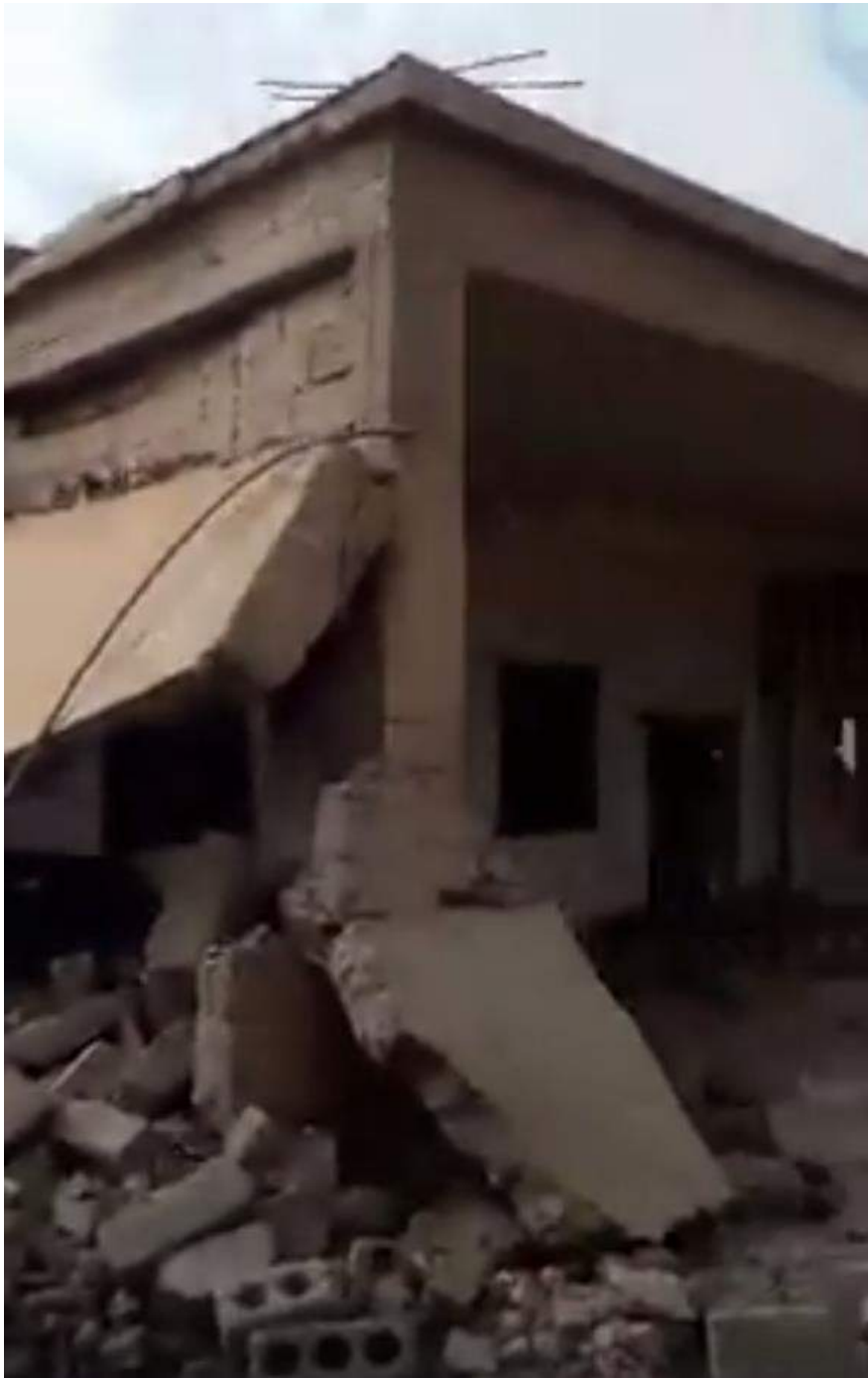
Damage to the northeast corner of mosque (al-Boukamal al-Mayadin al-Balad/November 29, 2017)
