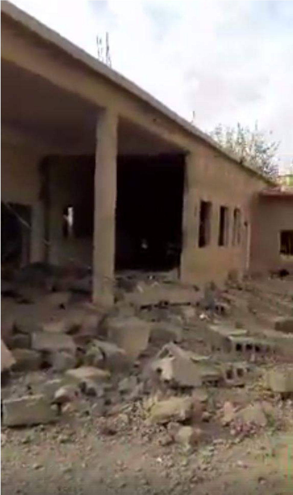
Damage to the northern section of mosque (al-Boukamal al-Mayadin al-Balad/November 29, 2017)
