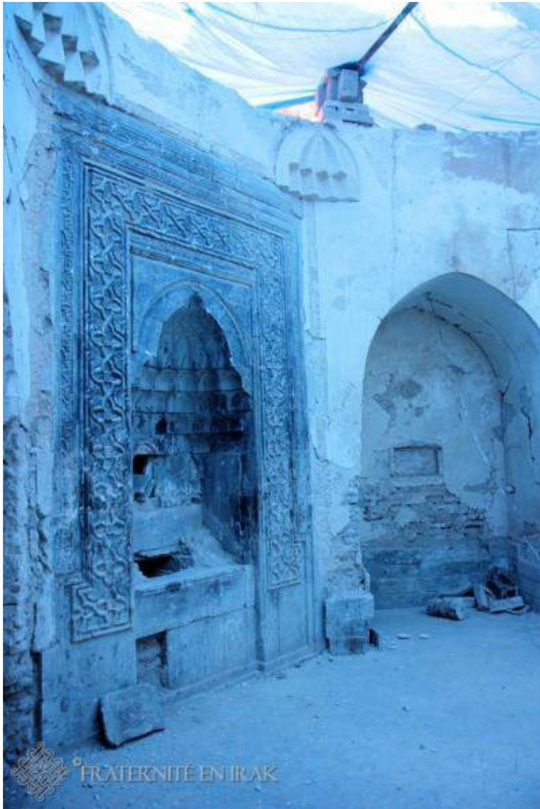
Restoration work begins on the niche containing the relics of Mar Behnam Monastery (Fraternité in Irak; October 27, 2017)
