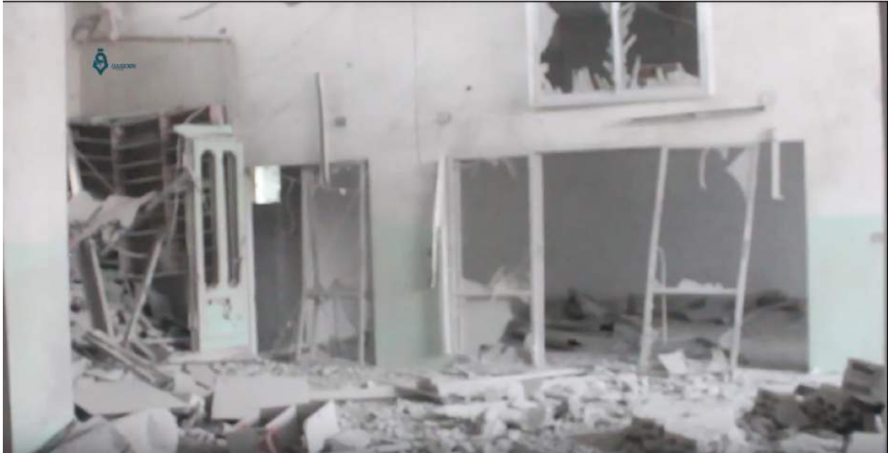
Video still of damage to the interior of al-Kabir Mosque (Qasioun News Agency; September 29, 2017)
