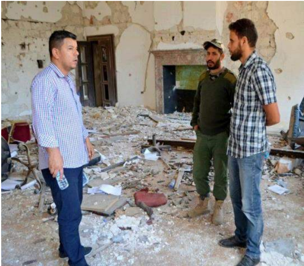
Damaged interior of the Qasr al Manar (Libyan Antiquities Authority; November 2, 2017)
