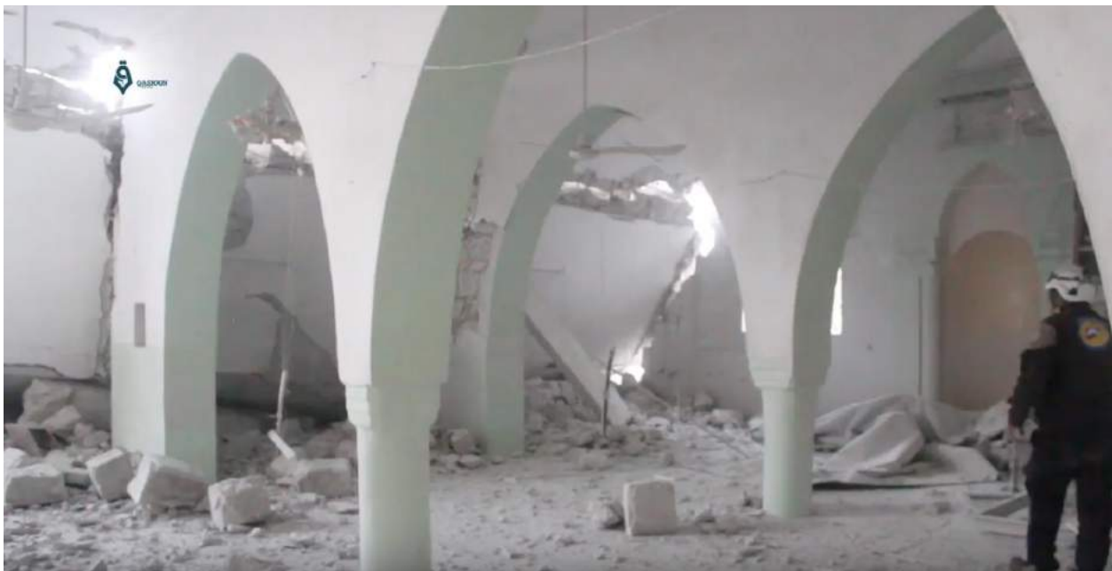
Video still of damage to the interior of al-Kabir Mosque (Qasioun News Agency; September 29, 2017)
