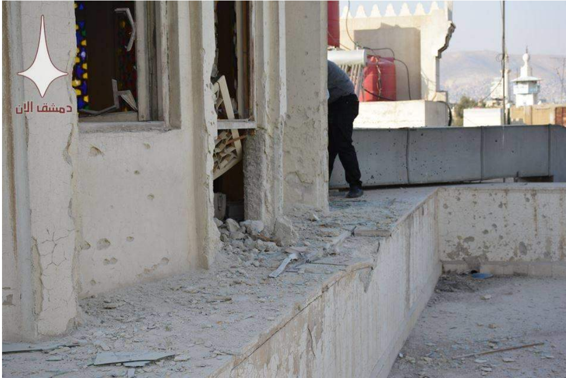
Damage to the dome of the mosque (Dimashq al-Aan; November 27, 2017)
