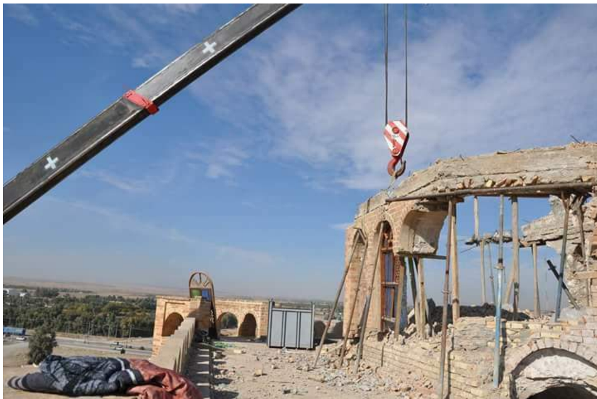
Antiquities department works to reconstruct damaged section of castle (Director-General of Antiquities; November 30, 2017)
