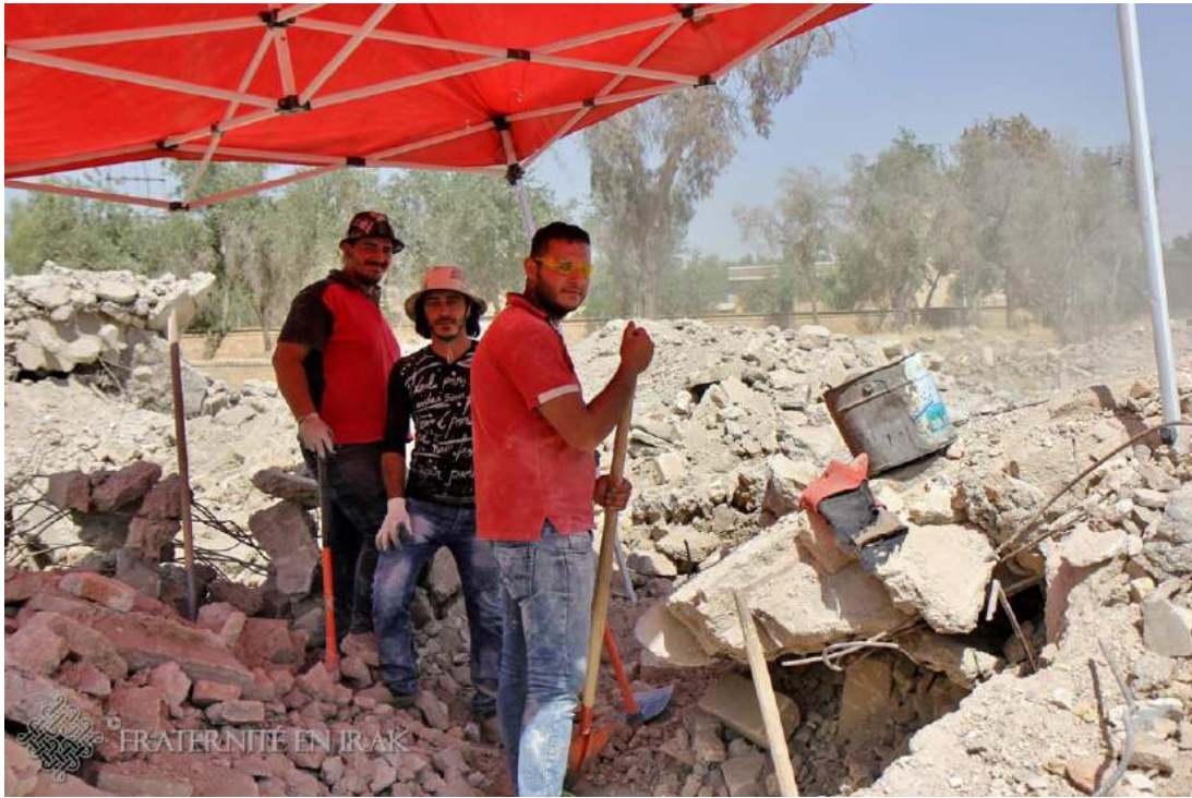
Workers sort and clear rubble during reconstruction of Mar Behnam Monastery (Fraternité in Irak; October 27, 2017)
