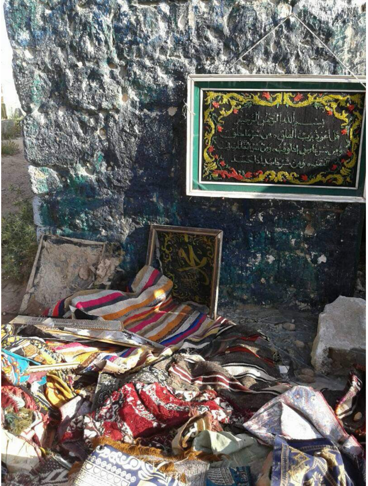
Vandalism of the exterior of Shrine of Sheikh Zaid, within contents of tomb removed (Private Twitter Account; May 18, 2018)
