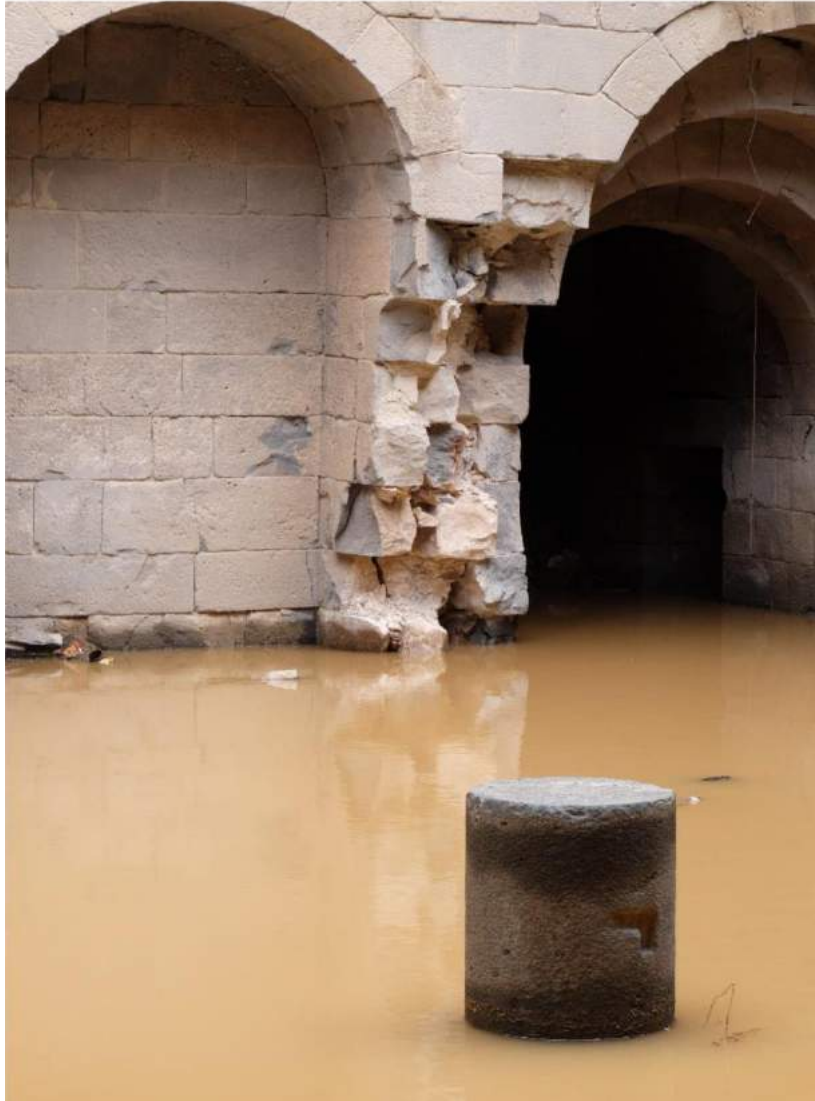
Water covers the destroyed parts of the west courtyard.
