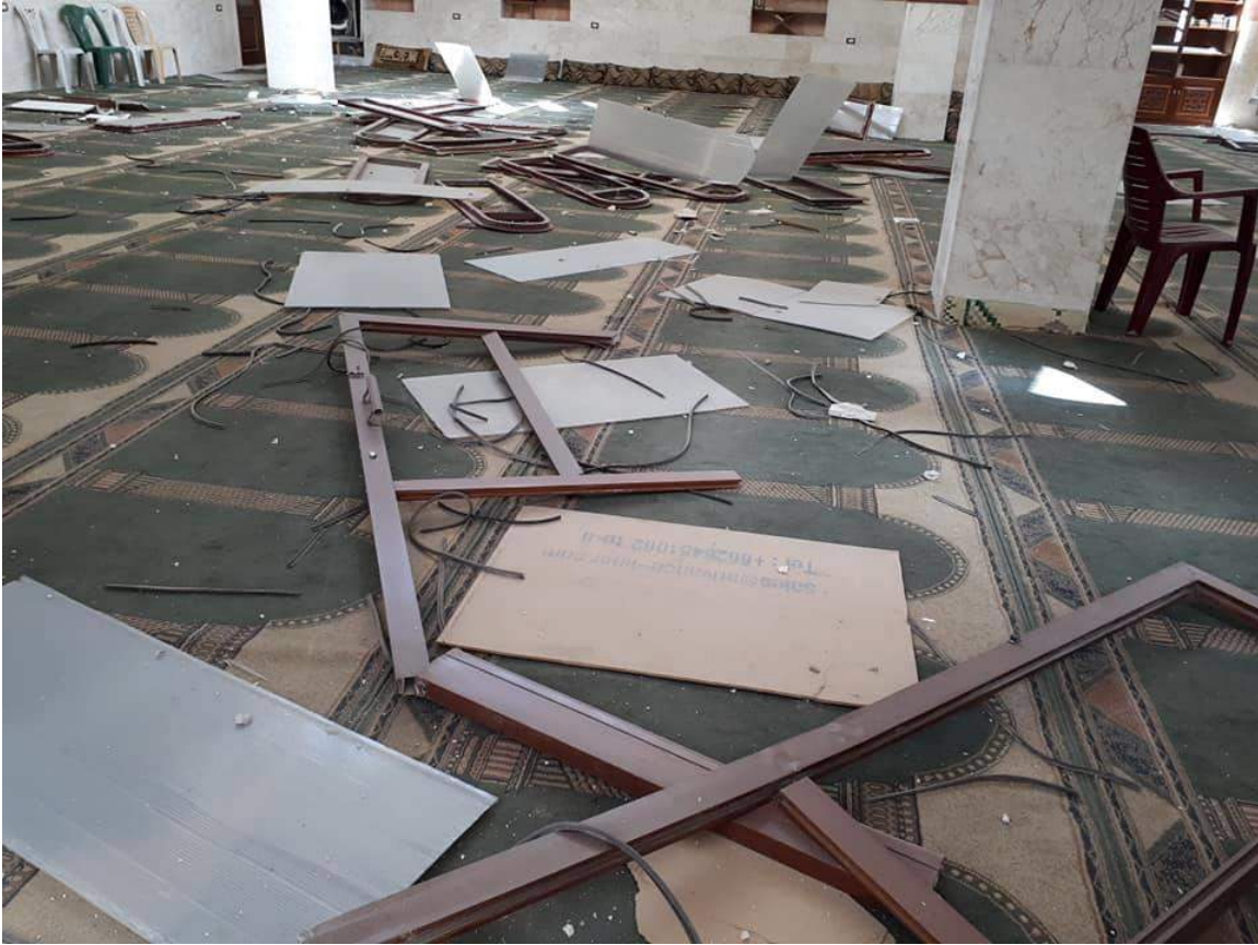
Damage to furniture in the interior of Hamza bin Abd al-Mutalleb Mosque (SNHR; May 6, 2018)
