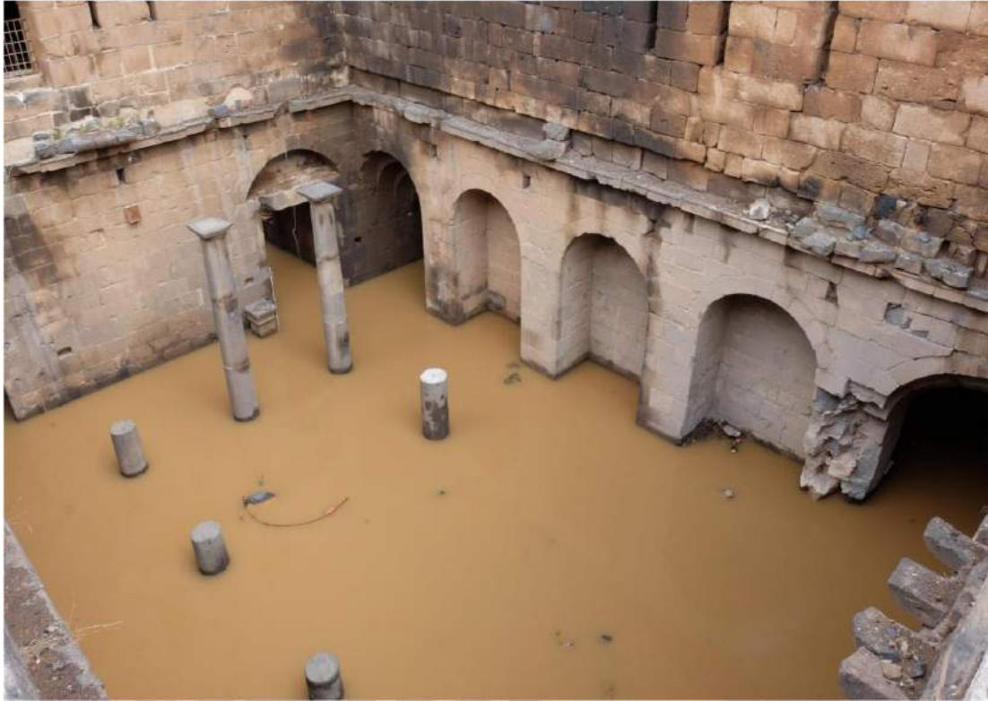
Another view of the west courtyard under water. Note the destruction caused by airstrikes.
