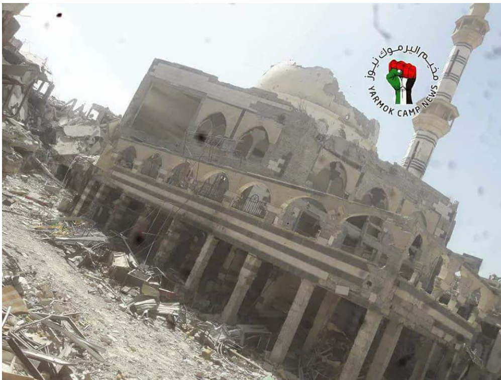
Damage to the Palestinian Mosque and the surrounding area, including the collapse of the dome (Private Twitter Account; May 11, 2018)
