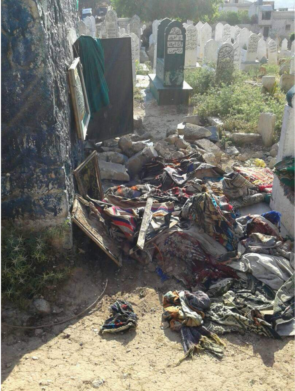
Vandalism of the exterior of Shrine of Sheikh Zaid (Private Twitter Account; May 18, 2018)
