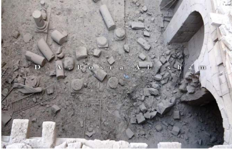
West courtyard after the airstrikes.
