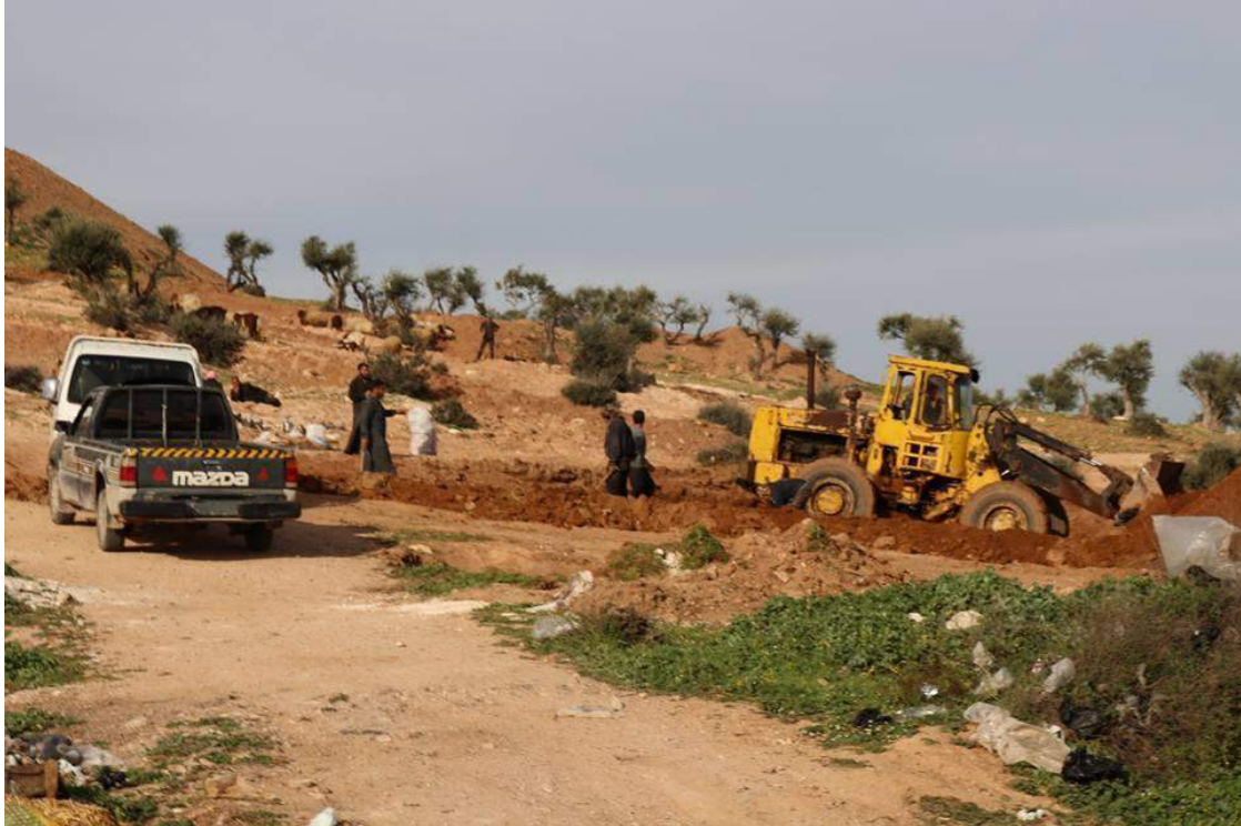
Bulldozer moving soil from around the base of Tell Danit (Ensemble Pour Les Antiquités; March 27, 2018)
