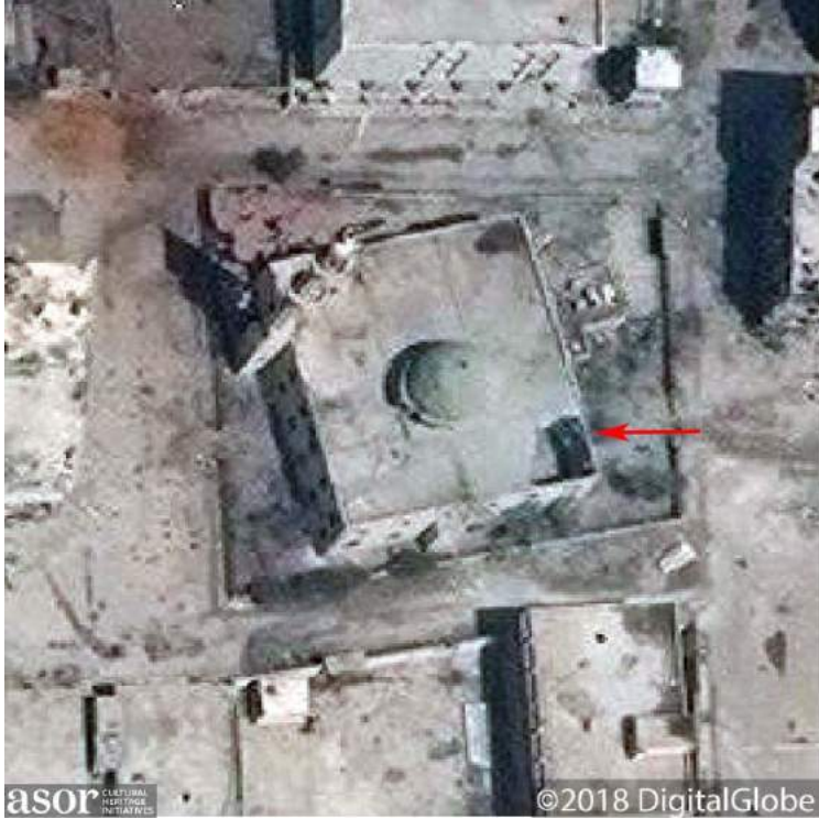
Initial damage to al-Zubair mosque with the collapse of the southeast part of the roof, indicated by a red arrow (DigitalGlobe NextView License; April 27, 2018)
