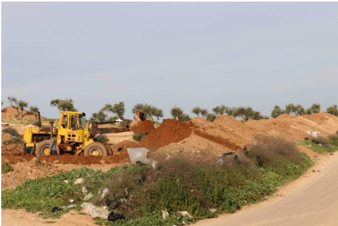
Bulldozer piling up soil for removal near the base of Tell Danit (Ensemble Pour Les Antiquités; March 27, 2018)
