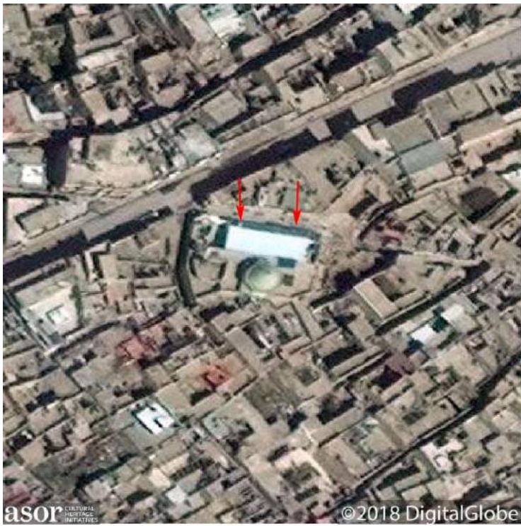
Red arrows indicate reconstruction to the mosque's roof (DigitalGlobe NextView License; March 12, 2018)
