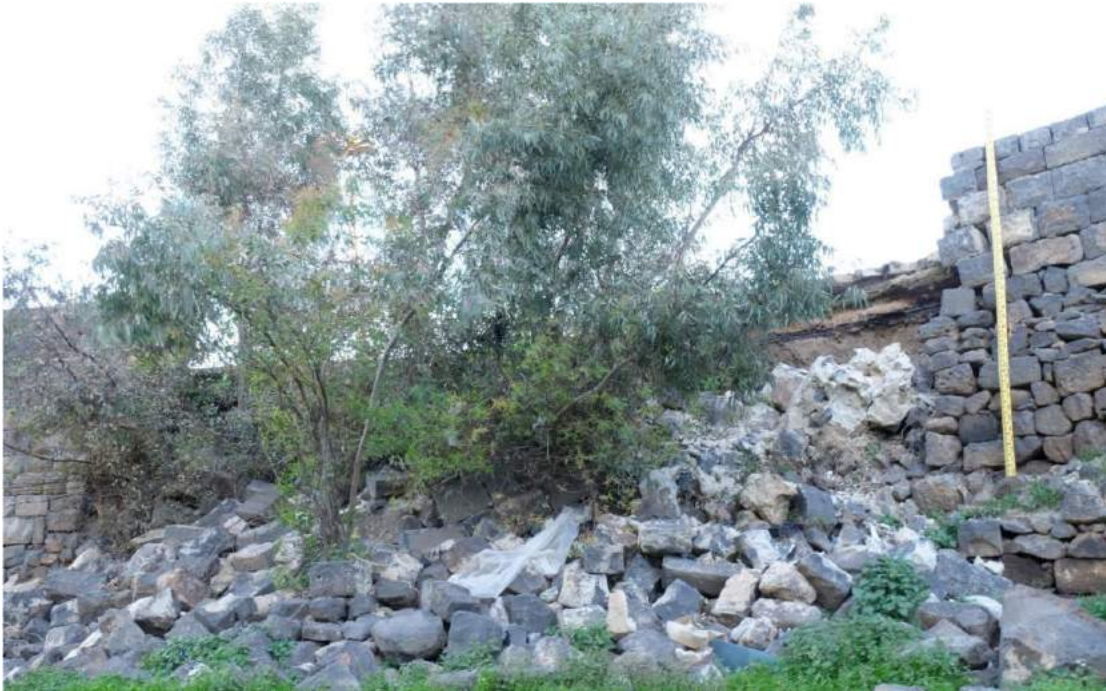
Images showing collapsed outer walls of the trench surrounding the citadel due to the massive floods
