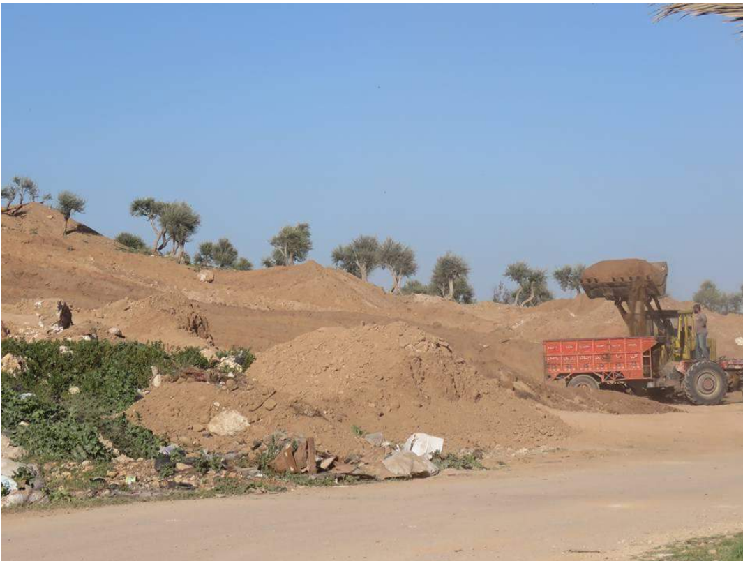
Bulldozer loading soil from Tell Danit onto truck for removal (Ensemble Pour Les Antiquités; March 27, 2018)
