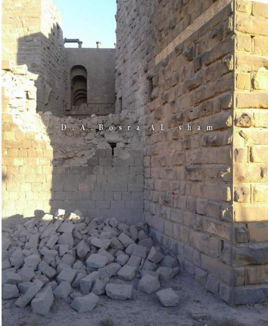
The citadel's western wall near the fifth tower is destroyed.
