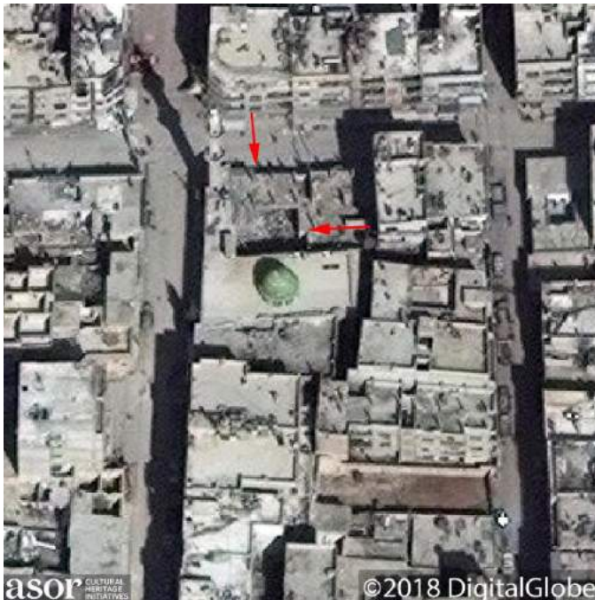
Partial collapse of the inner roof of al-Sleiq Mosque is indicated by the red arrows (DigitalGlobe NextView License; March 1, 2018)
