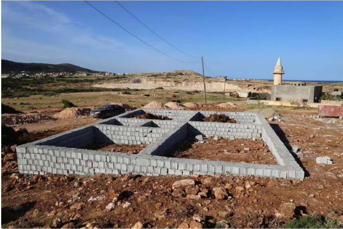
New foundations have been laid in concrete block on top of the archaeological site (DoA Shahat; March 19, 2018)
