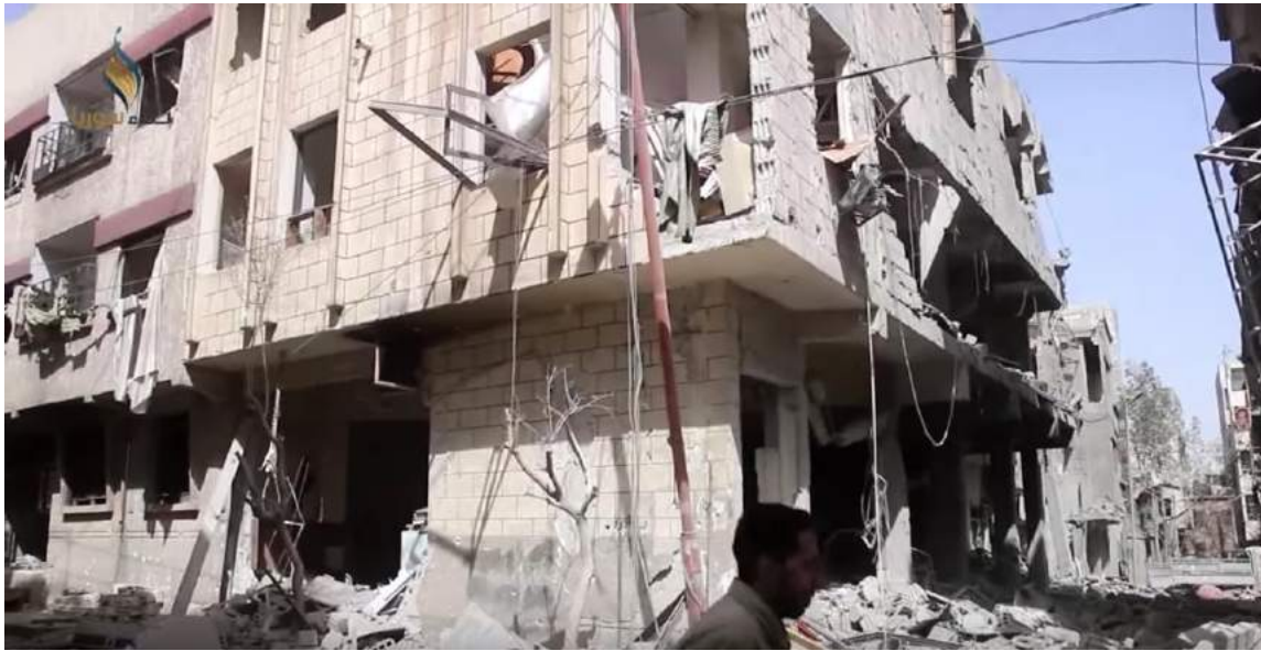
Video still showing severe damage to exterior of al-Mahmoud Mosque (Damascus Media Center; March 19, 2018)
