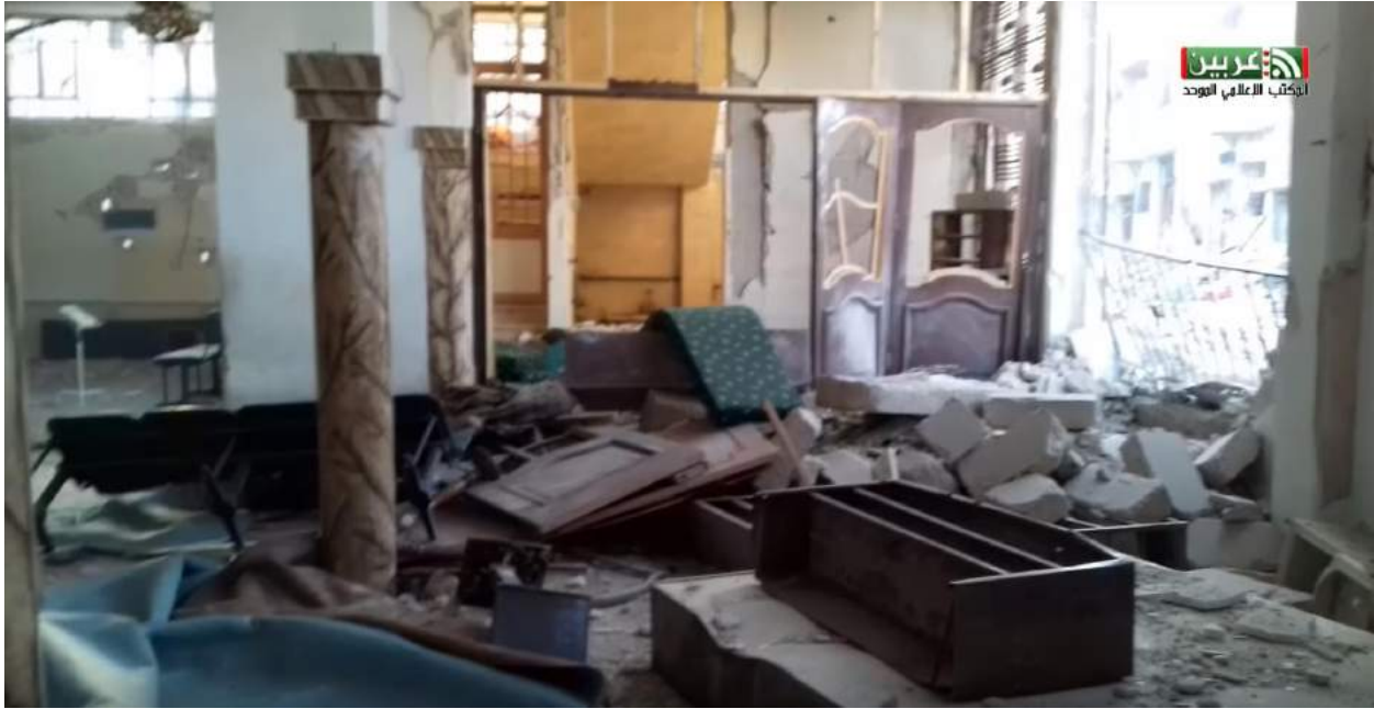
Video still showing severe damage to the interior of al-Kabir Mosque (Unified Media Office in Arbin; March 13, 2018)
