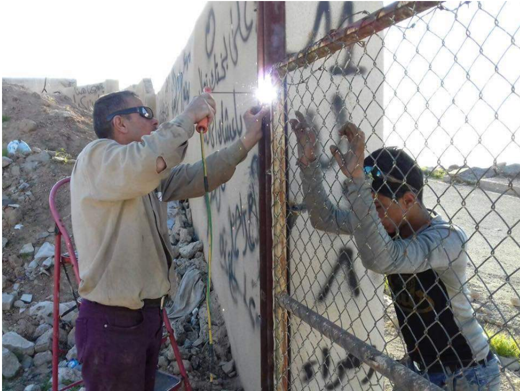
A view of the installation of the gate at the Nebi Yunus Mosque Complex (Ziusudra; March 27, 2018)
