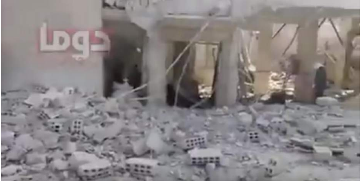
A video still shows severe damage to the exterior of al-Sleiq Mosque (SNHR; March 12, 2018)
