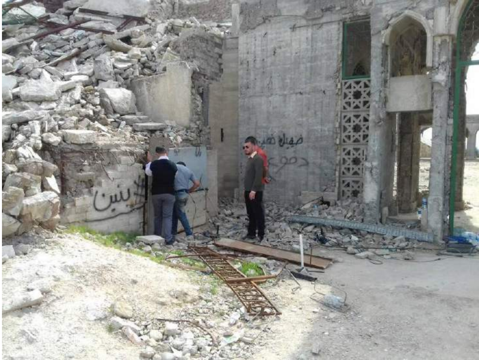
The installation of one of the blockings at the Nebi Yunus Mosque Complex (Ziusudra; March 27, 2018)
