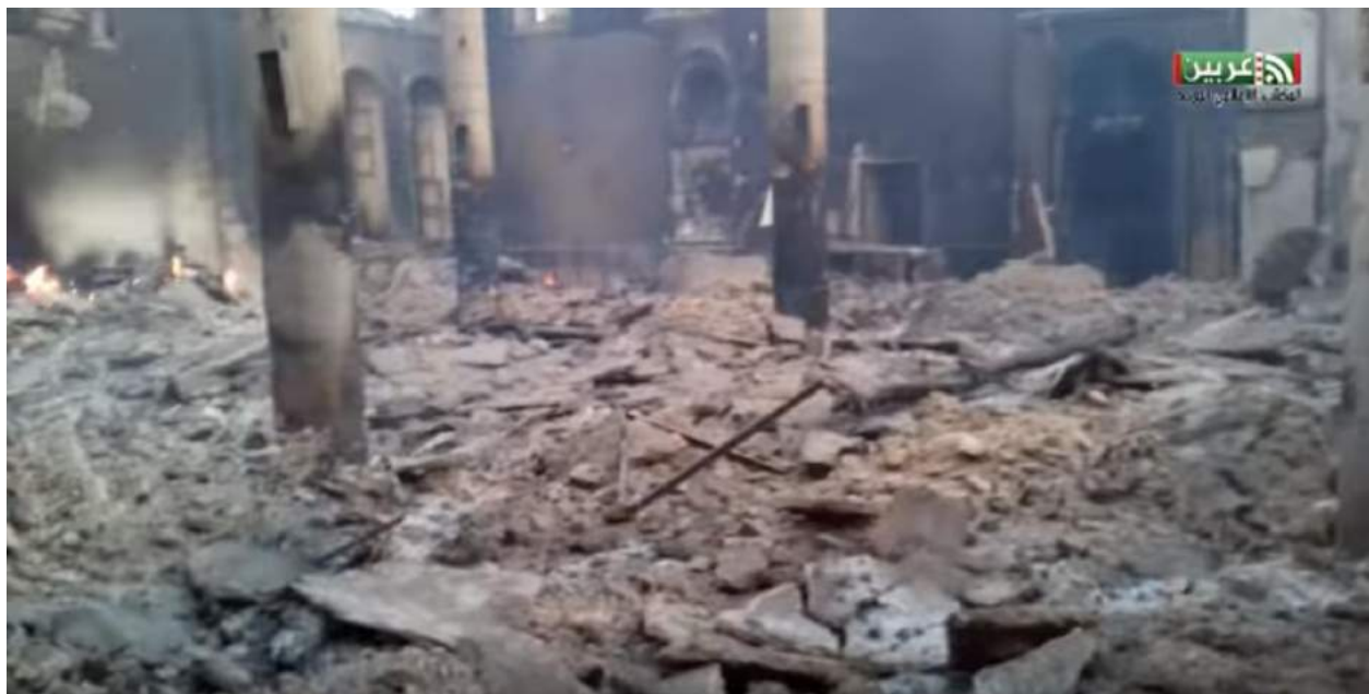
Video still showing fire in and severe damage to the interior of al-Kabir Mosque (Unified Media Office in Arbin; March 13, 2018)
