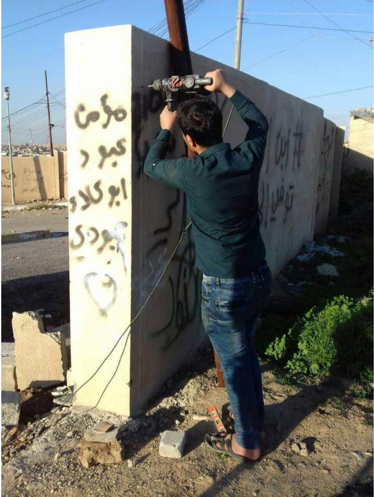
A view of the gate installation process at the Nebi Yunus Mosque Complex (Ziusudra; March 27, 2018)
