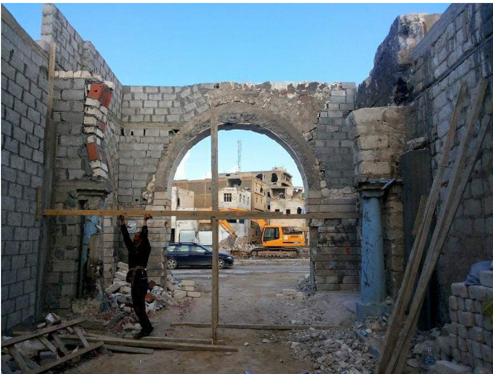
Works progress to re-erect arches and stabilize others with infill of concrete masonry (Private Facebook Account; March 28, 2018)
