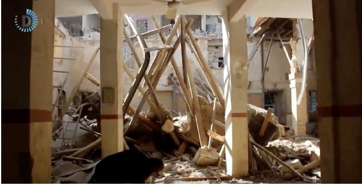
A video still shows severe damage to the interior of al-Sleiq Mosque (SNHR; March 12, 2018)
