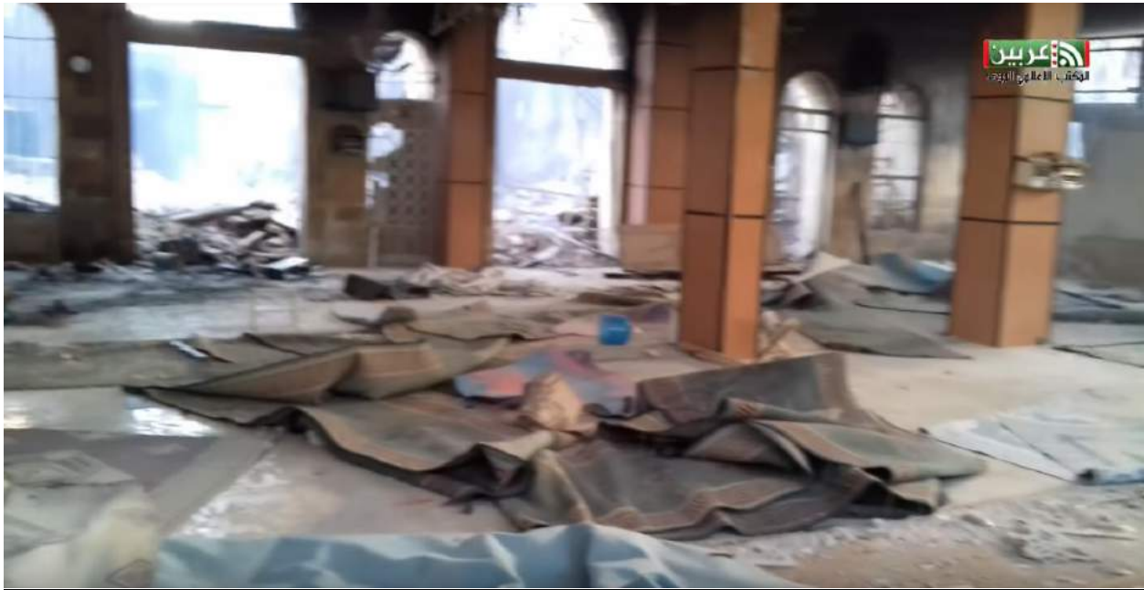
Video still showing severe damage to the interior of al-Kabir Mosque (Unified Media Office in Arbin; March 13, 2018)
