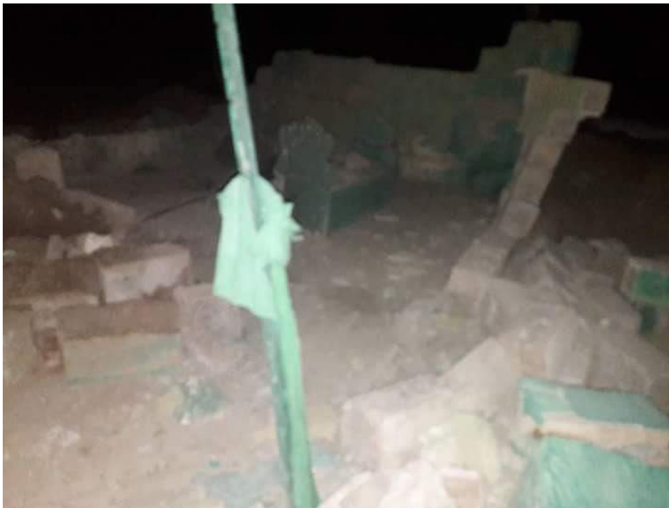
The toppled walls of Sayed Rebar Shrine, seen from the east (Private Twitter Account; March 21, 2018)
