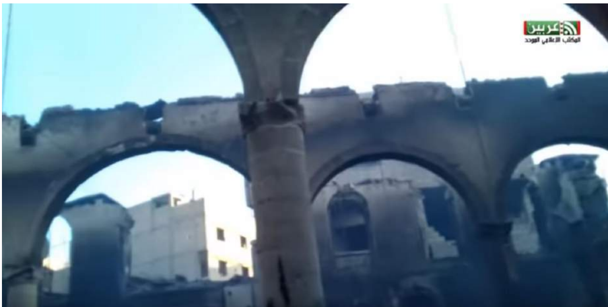
Video still showing severe damage to al-Kabir Mosque (Unified Media Office in Arbin; March 13, 2018)
