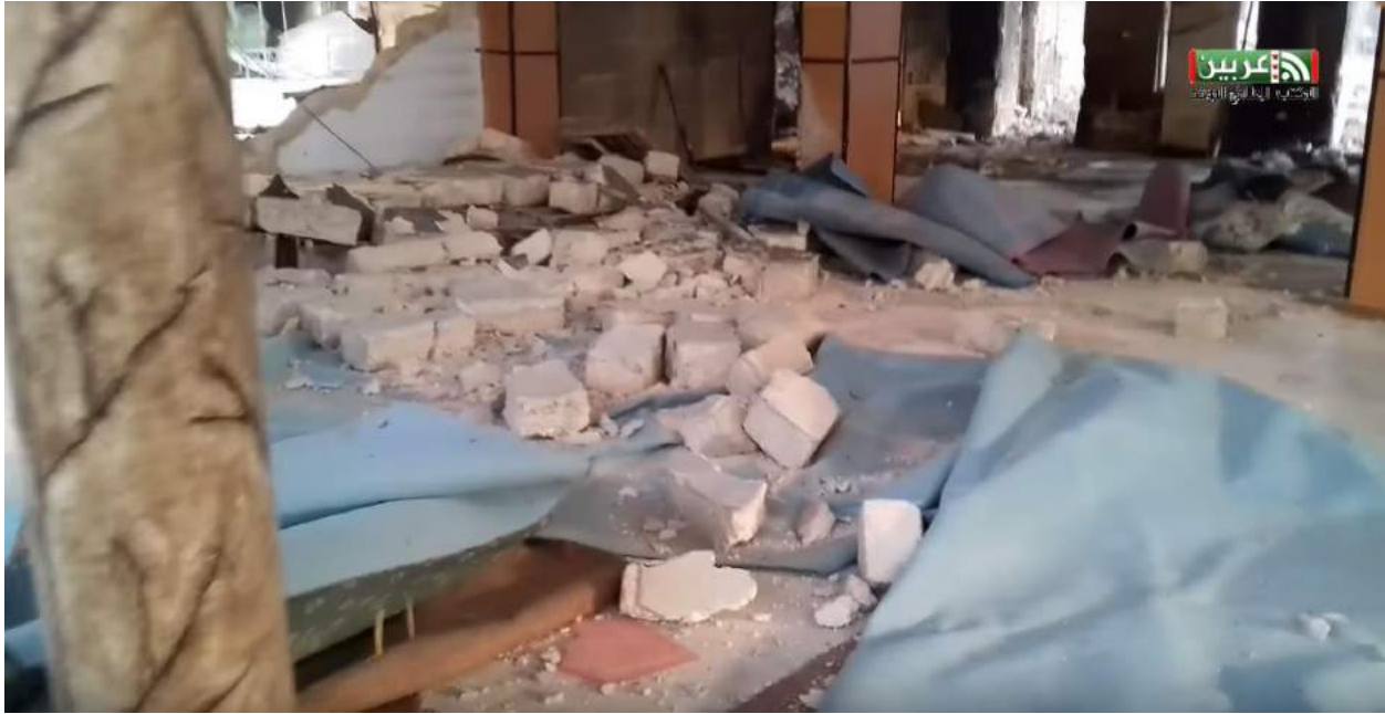
Video still showing severe damage to the interior of al-Kabir Mosque (Unified Media Office in Arbin; March 13, 2018)
