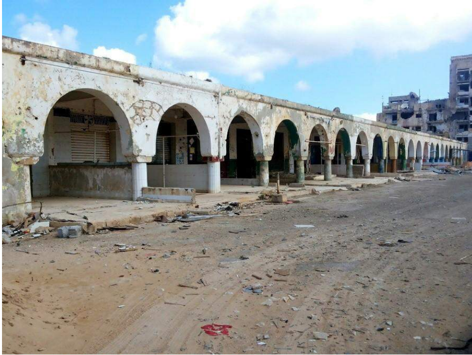
For some portions of the Souq al Baladi, the damage was less severe and necessary repairs are largely cosmetic (Private Facebook Account; March 28, 2018)
