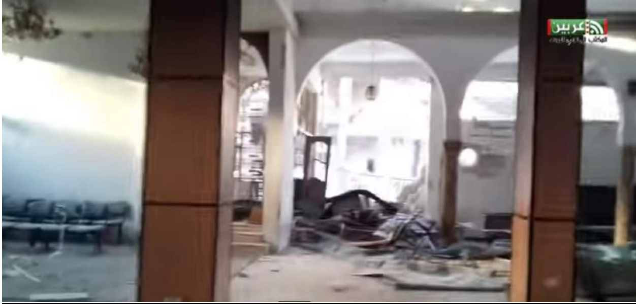
Video still showing damage to the interior of al-Kabir Mosque (Unified Media Office in Arbin; March 13, 2018)
