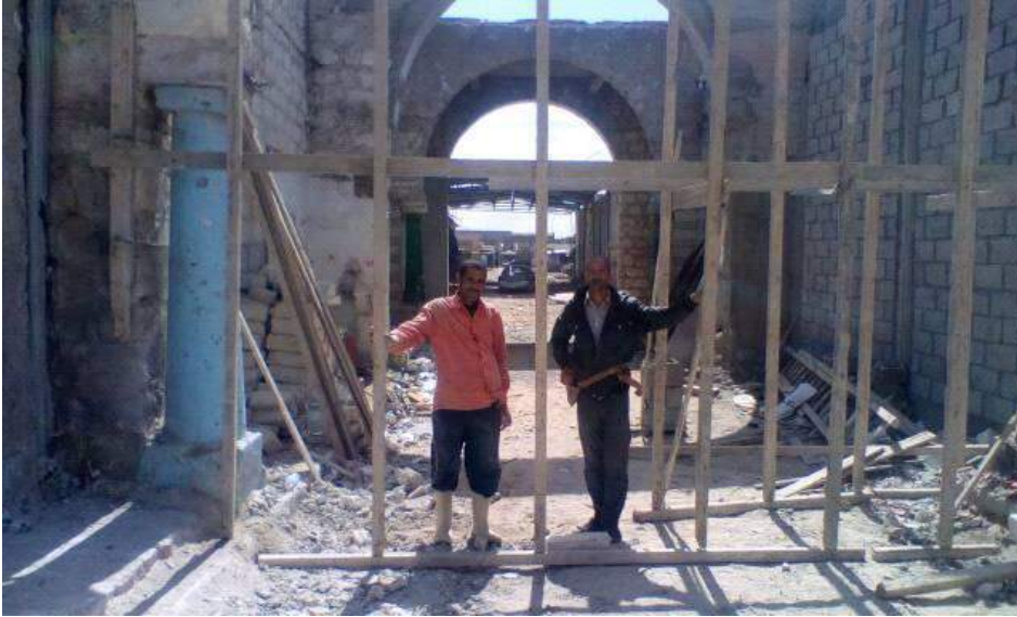
Members of DoA Benghazi pose by scaffolding erected to stabilize portions of this historic entryway (Private Facebook Account; March 28, 2018)
