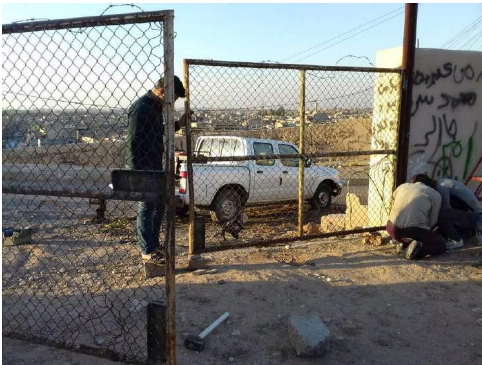
The finishing touches on the gate installation at the Nebi Yunus Mosque Complex (Ziusudra; March 27, 2018)
