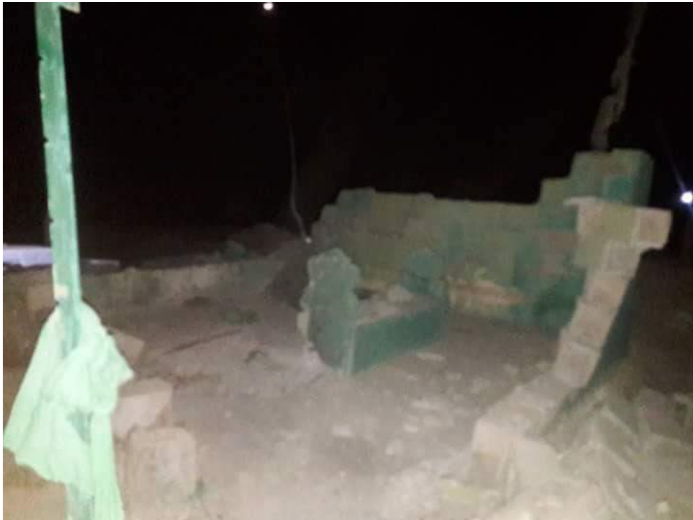
The interior of Sayed Rebar Shrine, seen from the east (Private Twitter Account; March 21, 2018)
