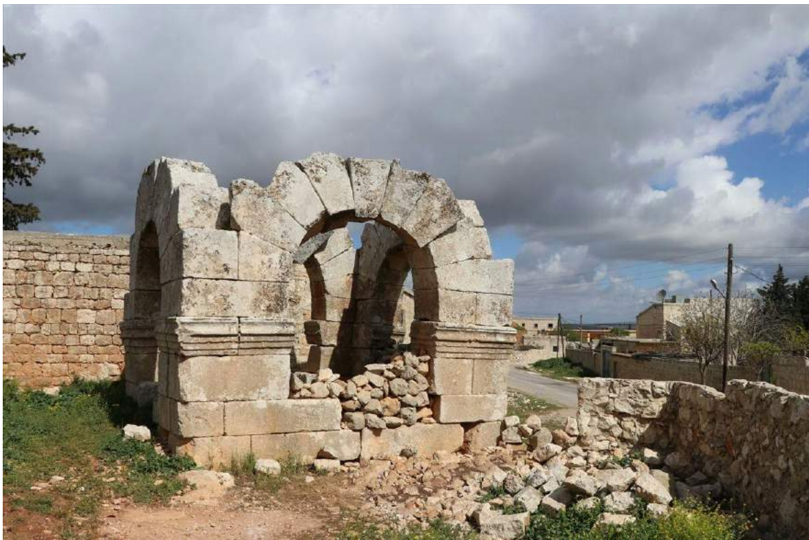
A tetrapylon at Barad. Multiple arches are in danger of collapsing (ASOR CHI Source; March 30, 2018)
