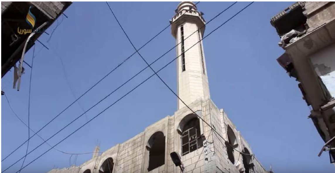
Video still showing severe damage to exterior of al-Mahmoud Mosque (Damascus Media Center; March 19, 2018)
