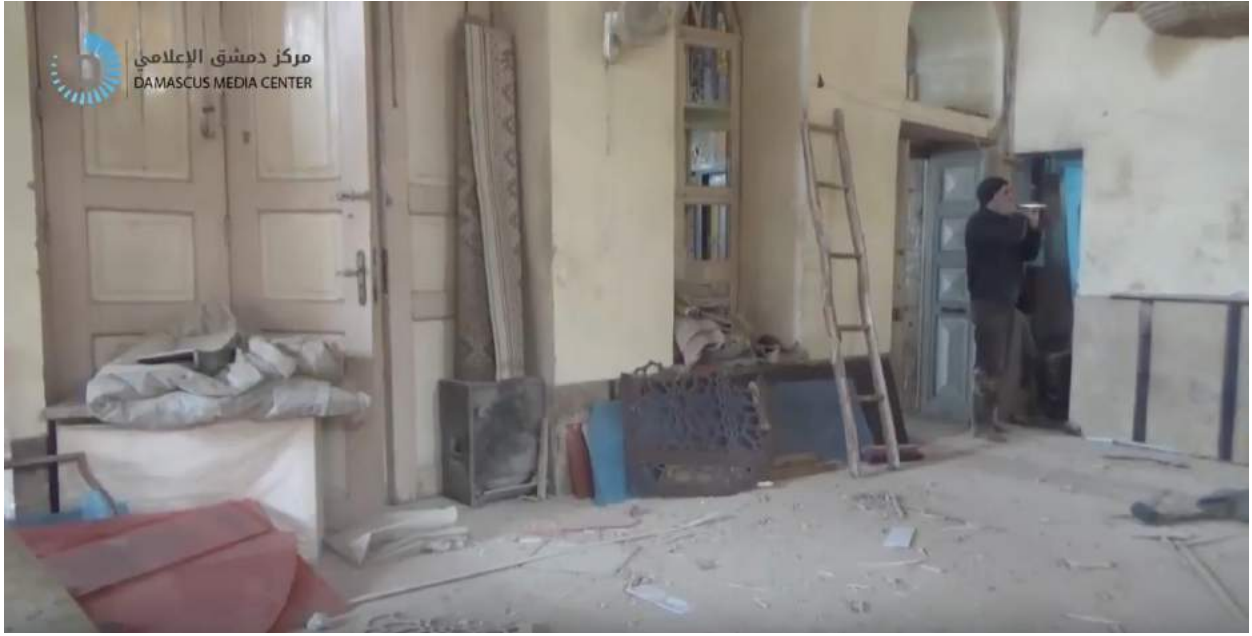
Video still of damage to al-Rahman Mosque interior (Damascus Media Center; January 22, 2018)
