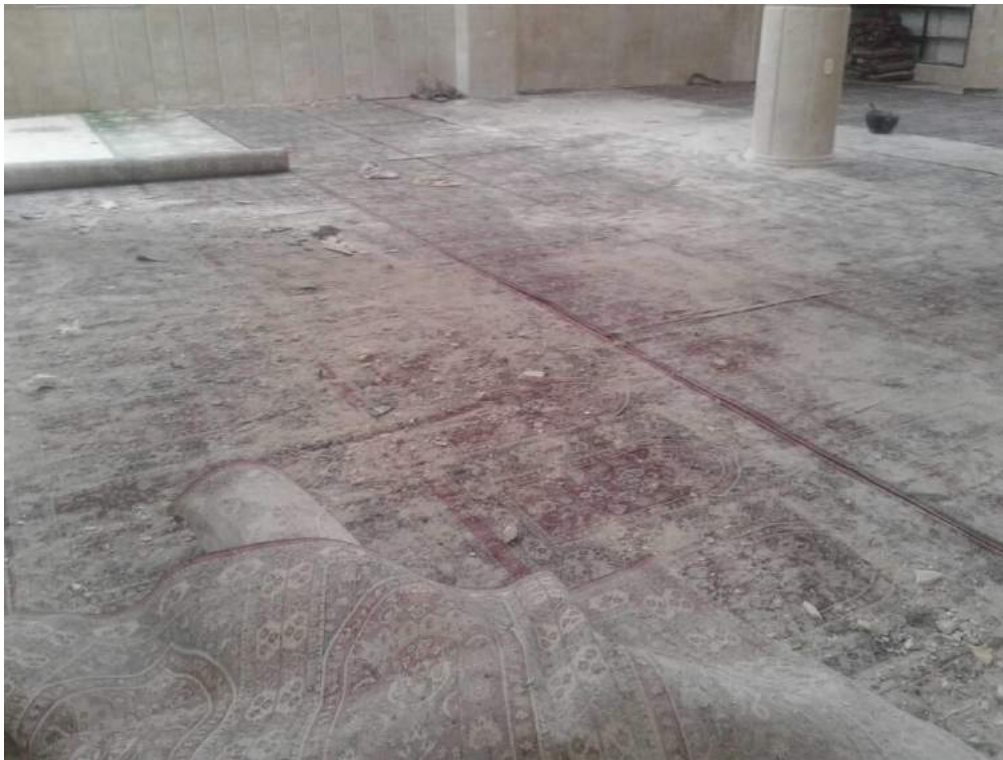
Damage to the interior of Uwais al-Qarni Mosque (ASOR CHI Source; January 4, 2018)
