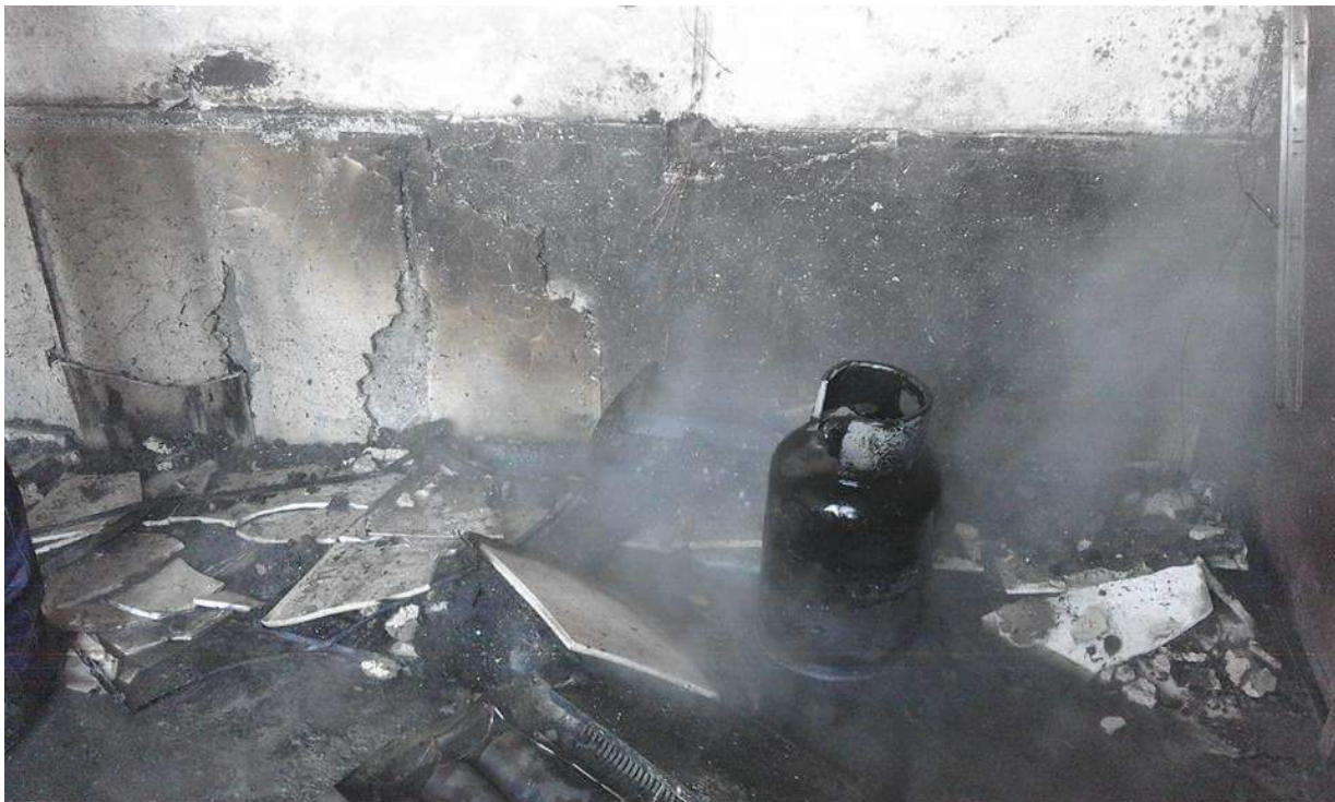
Fire damage seen in interior of Kaab bin Malik Mosque (Al-Zahra Neighborhood News Network; January 29, 2018)
