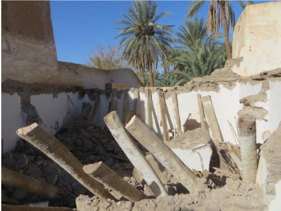
A structure in Ghadames collapsed due to rain and lack of maintenance (Mahmoud Hadia, December 27, 2017)
