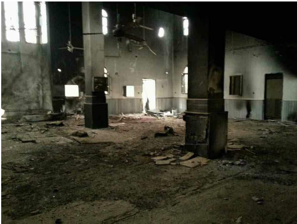
Damage to the interior of Khalid bin Walid Mosque, including evidence of fire damage (Euphrates Post; January 23, 2018)
