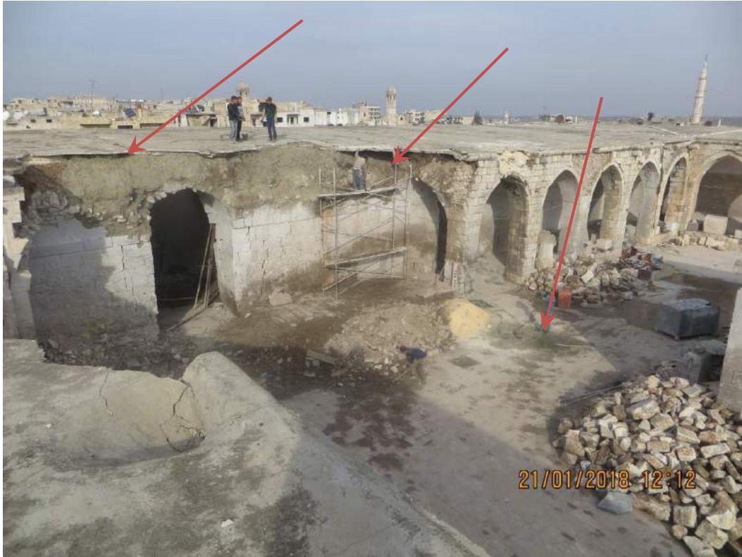
Repair work is ongoing to prevent deterioration of damaged areas from environmental conditions (TDA-HPI; January 21, 2018)
