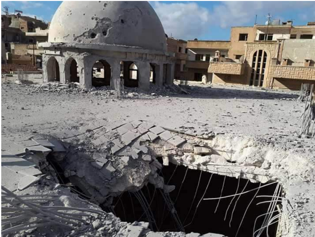
A hole in the roof of Uwais al-Qarni Mosque (Al Maara Media Center; January 2, 2018)
