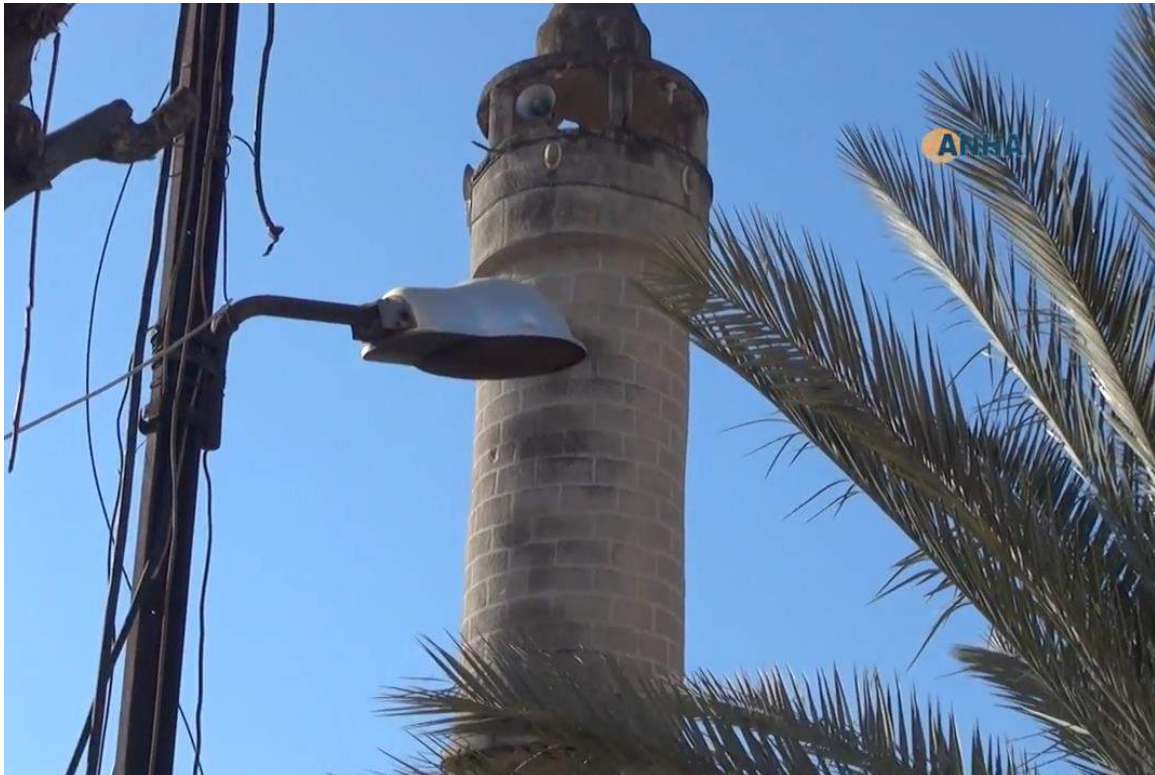
Video still of the minaret, with possible evidence of smoke damage, at Salah al-Din al-Ayoubi Mosque (ANHA; January 29, 2018)
