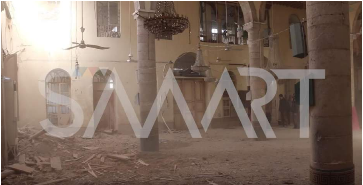
Video still of damage and debris in interior of al-Kabir Mosque (SMART News Agency; January 23, 2018)
