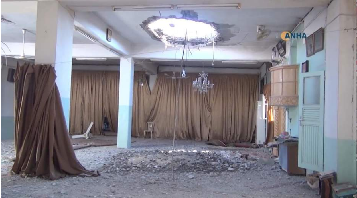
Video still of damage to the roof of Salah al-Din al-Ayoubi Mosque (ANHA; January 29, 2018)
