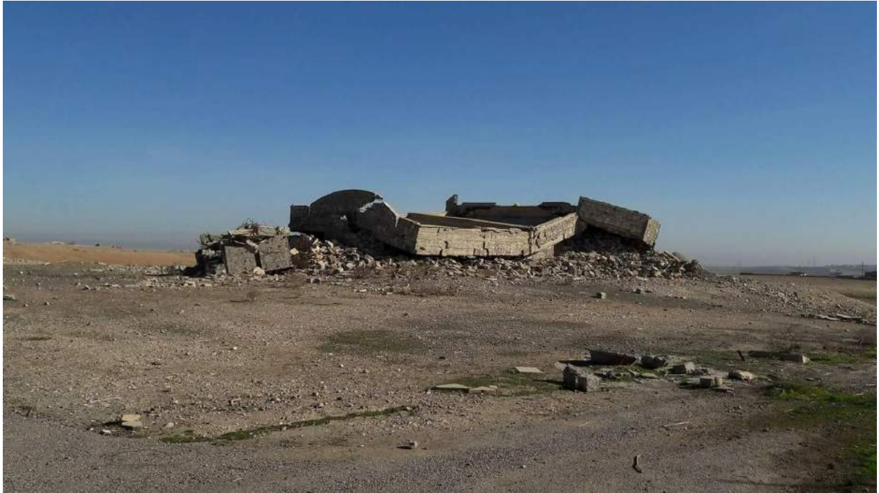
A destroyed structure near the entrance to the Christian section of Wadi 'Ikab Cemetery (This is Christian Iraq/Facebook; January 16, 2018)
