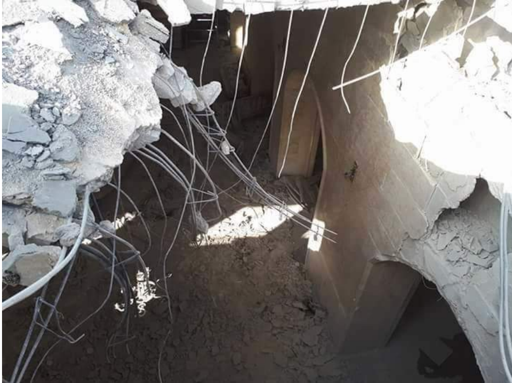
A hole in the roof and debris in the interior of Uwais al-Qarni Mosque (Al Maara Media Center; January 2, 2018)
