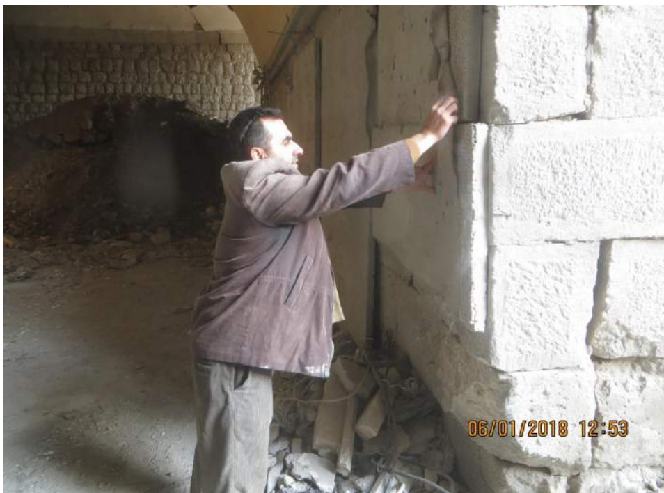
A worker assesses the damage and take measurements (TDA-HPI; January 6, 2018)
