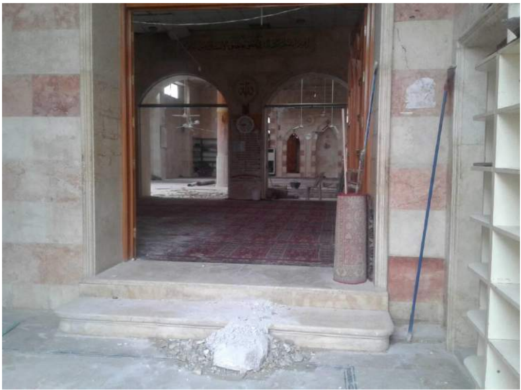
Damage to the interior of Uwais al-Qarni Mosque (ASOR CHI Source; January 4, 2018)
