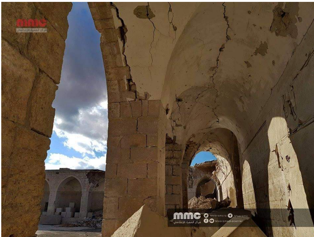
Damage to northern arcade in interior courtyard of al-Ma'arra Museum (Maara Media Center/Twitter; January 2, 2018)
