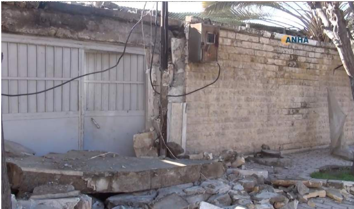
Video still of the exterior of Salah al-Din al-Ayoubi Mosque with evidence of recent damage (ANHA; January 29, 2018)
