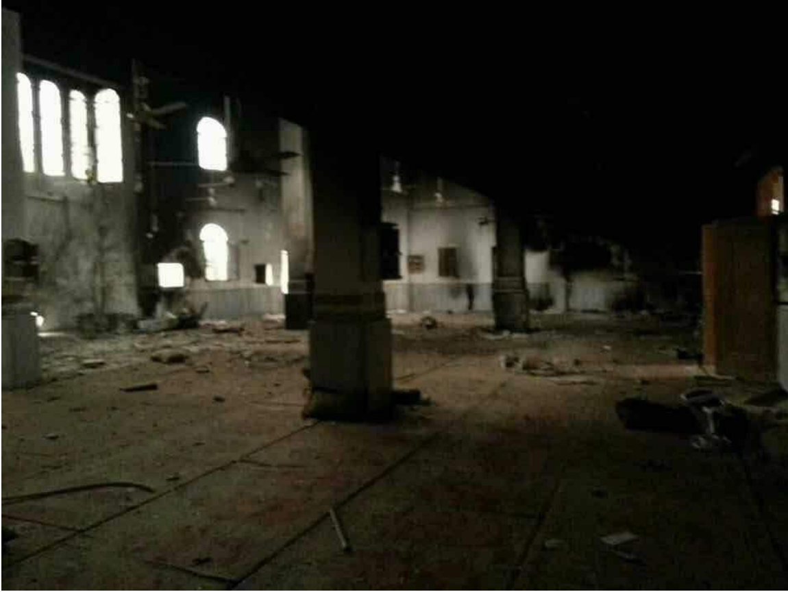
Damage to the interior of Khalid bin Walid Mosque, including evidence of fire damage (Euphrates Post; January 23, 2018)
