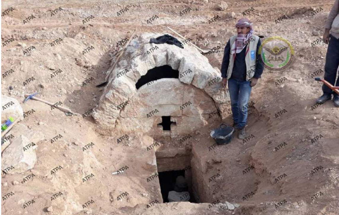
The ATPA conducts excavation and restoration work at al-Farahia Byzantine tomb (ATPA; January 4, 2018)
