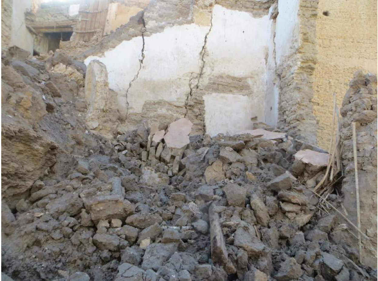
Residents have been relocated from the Old City of Ghadames, making it difficult to detect problems early, and harder to maintain the site as a whole (Mahmoud Hadia, December 27, 2017)
