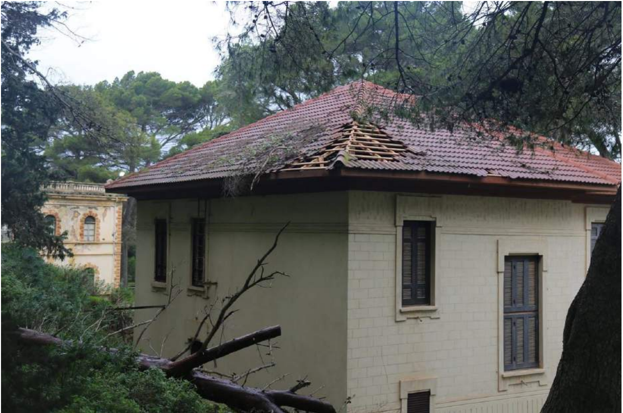
A view of the damaged section of the roof (DoA Shahat; January 4, 2018)
