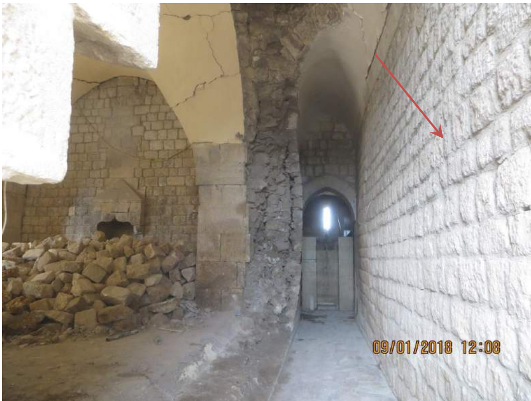
The wall previously dismantled and rebuilt, with the support of ASOR CHI was not affected by the missile strike (TDA-HPI; January 9, 2018)
