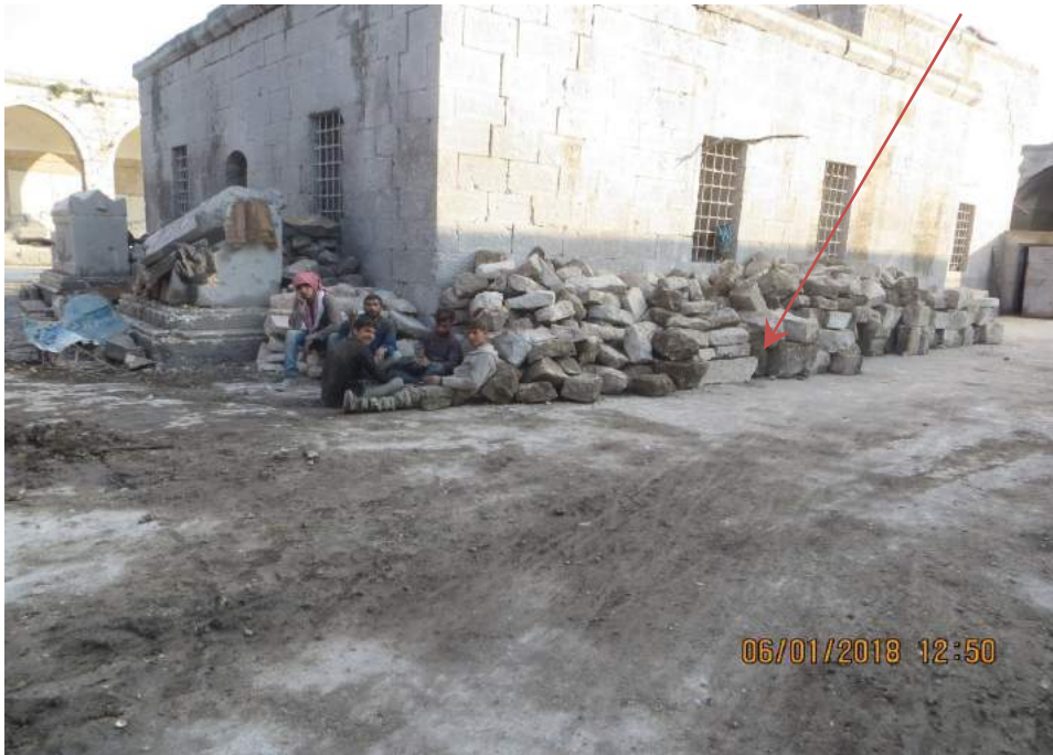
Workers gathered and sorted collapsed masonry in the central courtyard (TDA-HPI; January 6, 2018)
