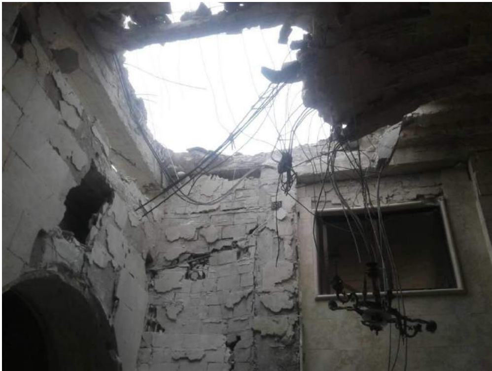
Damage to the interior of Uwais al-Qarni Mosque (ASOR CHI Source; January 4, 2018)
