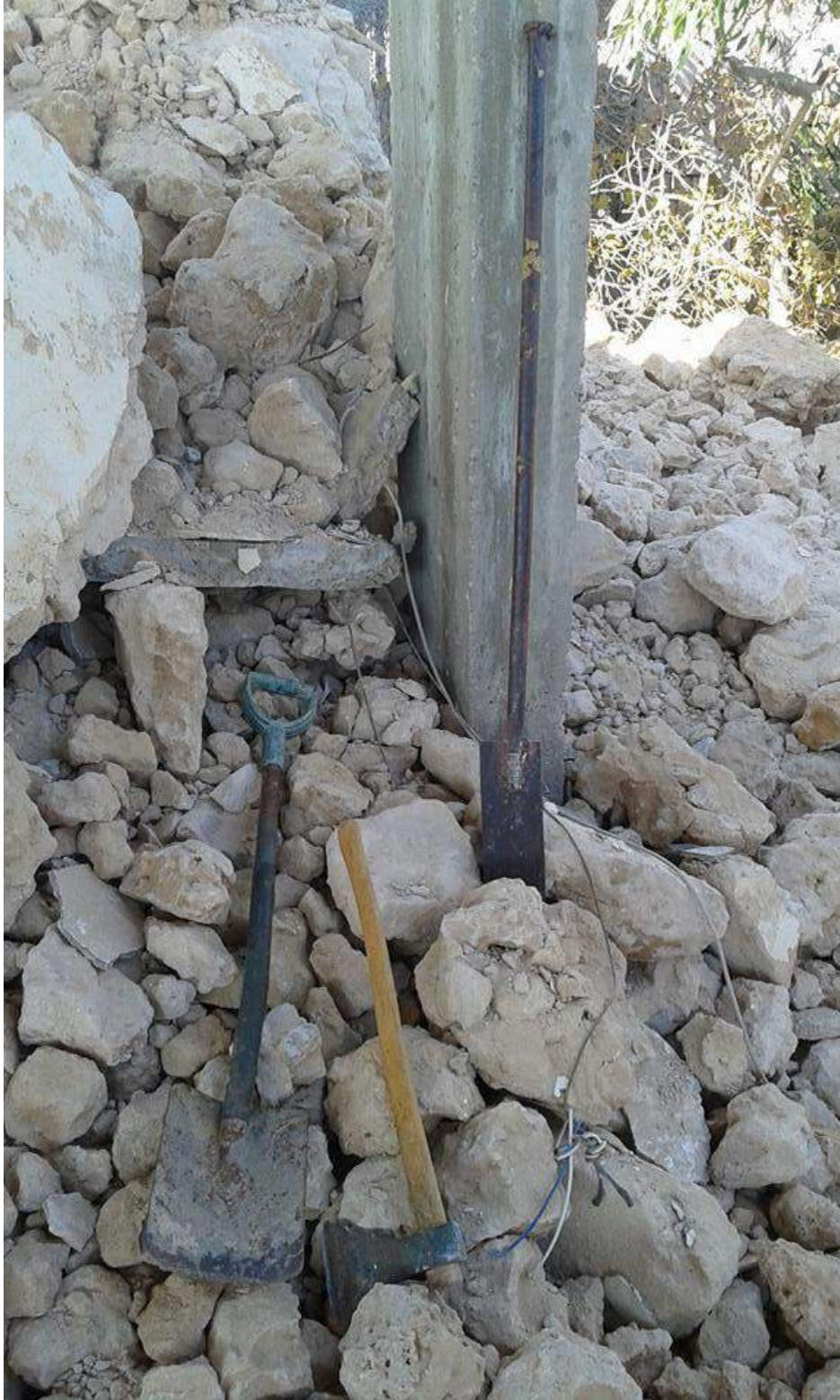
Image of tools used in demolition of the Shrine of Sheikh Muhammad ibn Marbat (Misratah Today; December 31, 2017)
