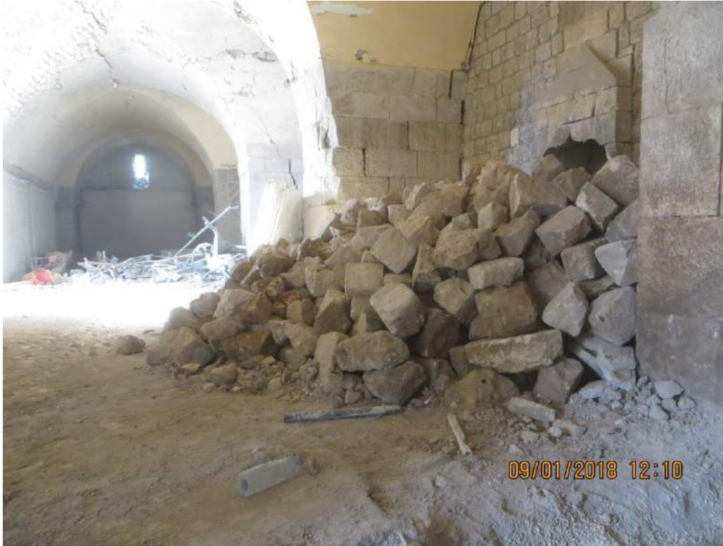
Workers gathered collapsed masonry (TDA-HPI; January 6, 2018)
