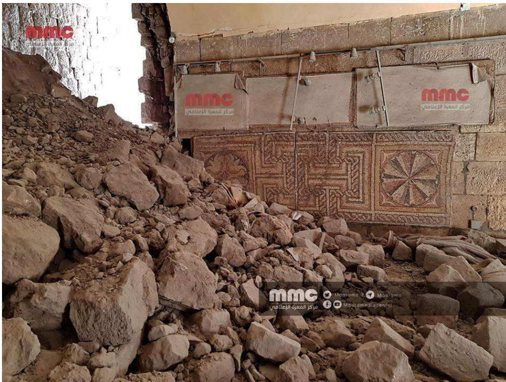
Collapsed section of arcade of al-Ma'arra Museum, with damaged Byzantine-era mosaic (Maara Media Center/Twitter; January 2, 2018)
