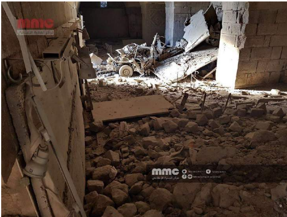
Damage to interior hallway of of al-Ma'arra Museum (Maara Media Center/Twitter; January 2, 2018)
