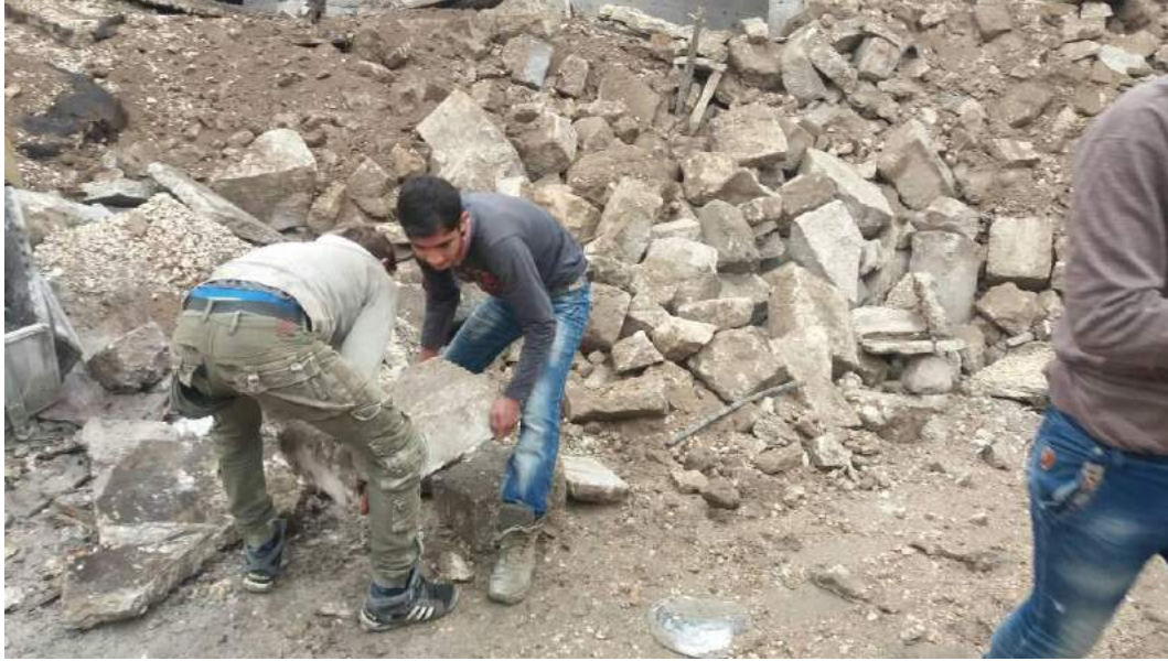
Workers sort rubble in the damaged northwest corner of museum (TDA-HPI; January 6, 2018)
