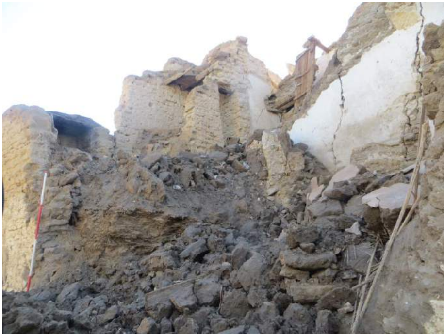
Many walls, long weakened by lack of maintenance, collapsed during a heavy rain at Ghadames (Mahmoud Hadia, December 27, 2017)
