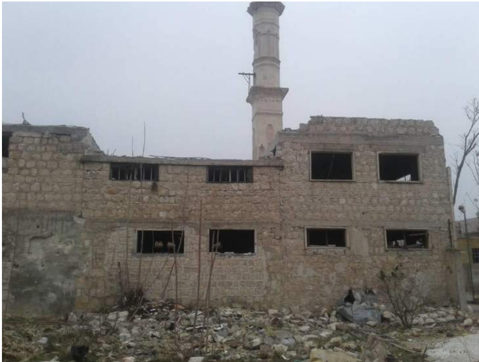
Damage to the exterior of Uwais al-Qarni Mosque (ASOR CHI Source; January 4, 2018)
