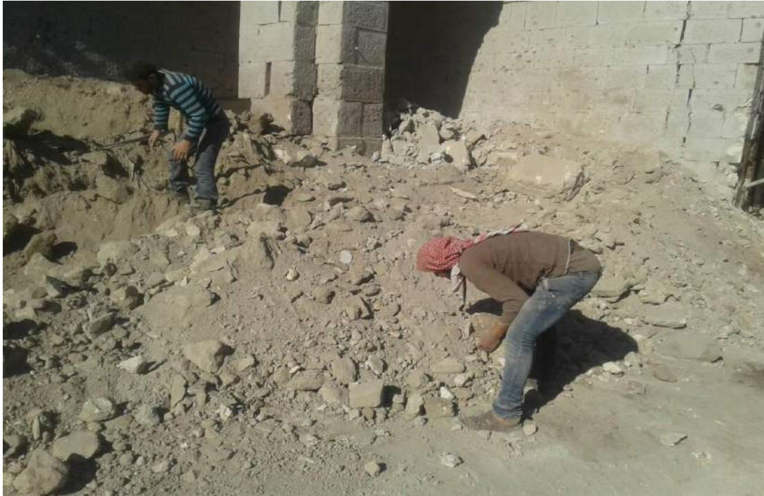
Workers sort through the rubble and collect fallen masonry in the damaged northwest corner (TDA-HPI; January 6, 2018)
