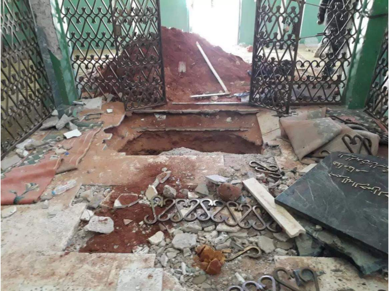
A view of the damage to the interior of the Mausoleum of al-Mahdi (Libyan Cloud News Agency; December 31, 2017)
