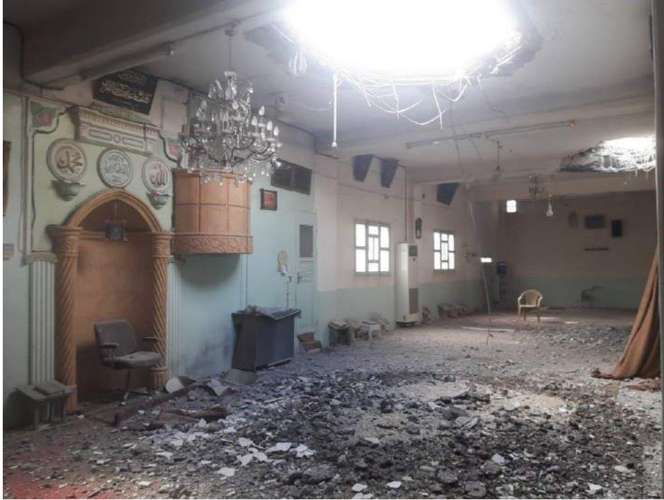
Damage to interior of Salah al-Din al-Ayoubi Mosque due to a large hole in the roof (SOHR; January 27, 2018)
