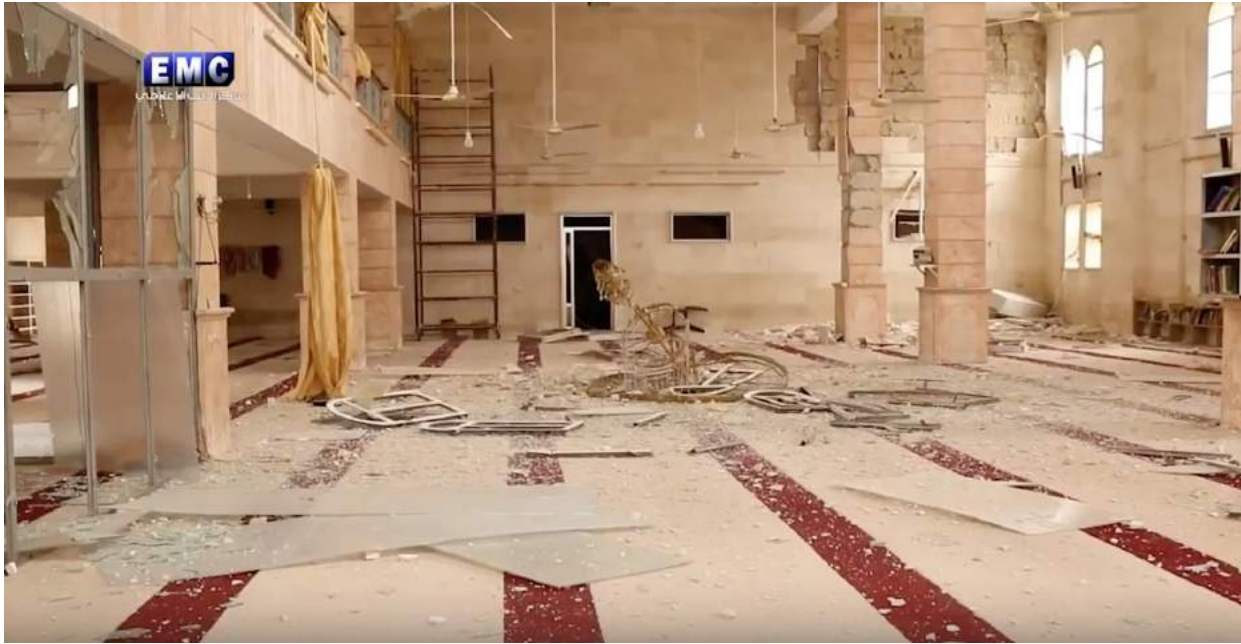
Video still of debris in the interior of al-Kabir Mosque (Edlib Media Center; January 4, 2018)
