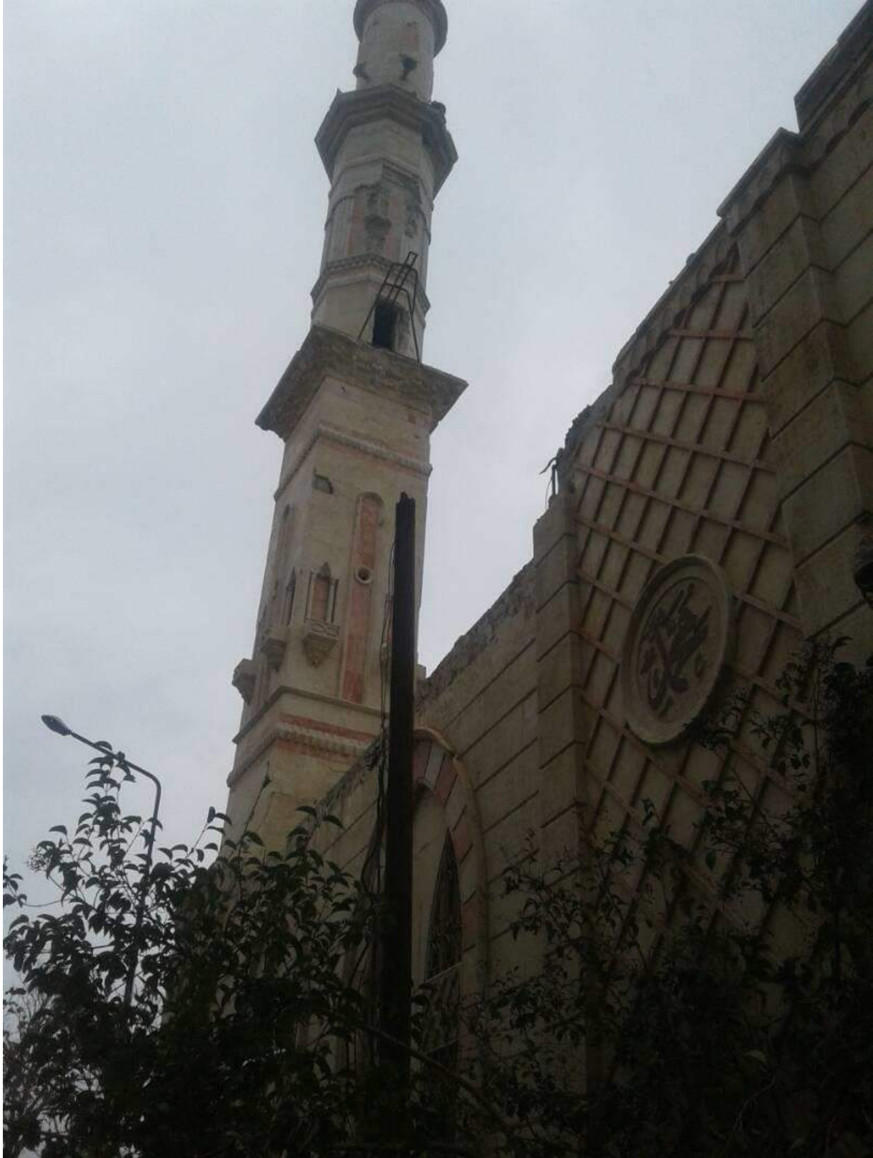
Minor damage to the minaret of Uwais al-Qarni Mosque (ASOR CHI Source; January 4, 2018)
