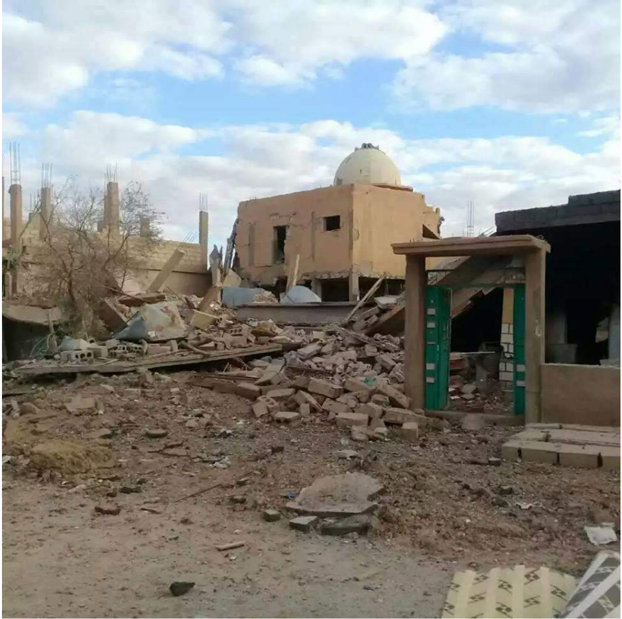
Damage to al-Farouq Mosque (Deir Ezzor 24; January 4, 2018)
