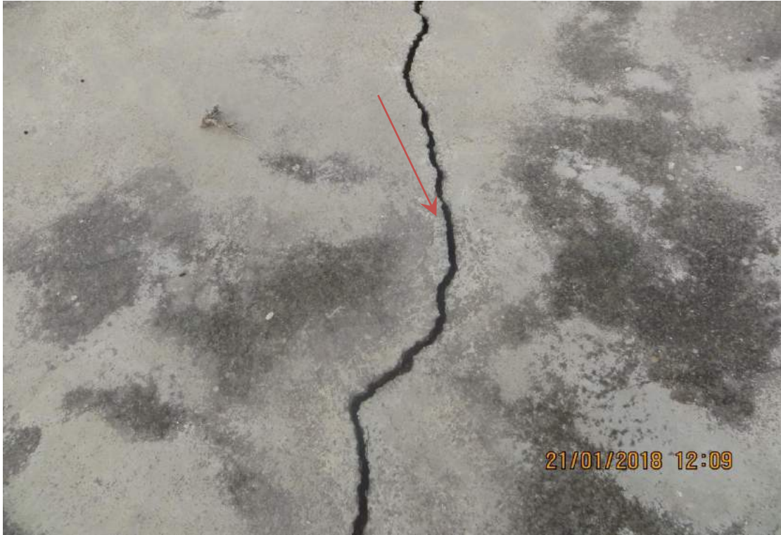
Crack prior to cement repair (TDA-HPI; January 21, 2018)
