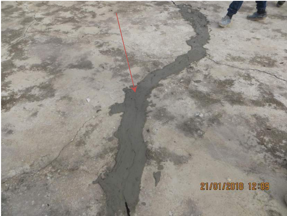
Crack following cement repair (TDA-HPI; January 21, 2018)
