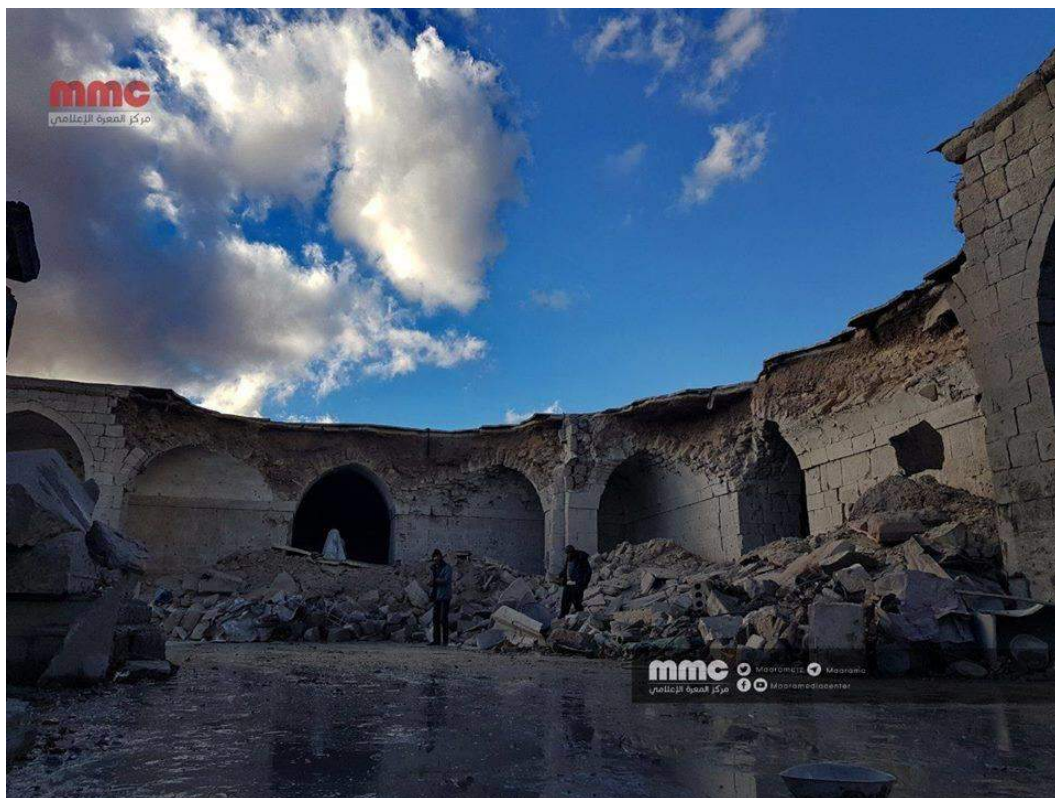
Damage to northeastern corner of arcade of al-Ma'arra Museum (Maara Media Center/Twitter; January 2, 2018)
