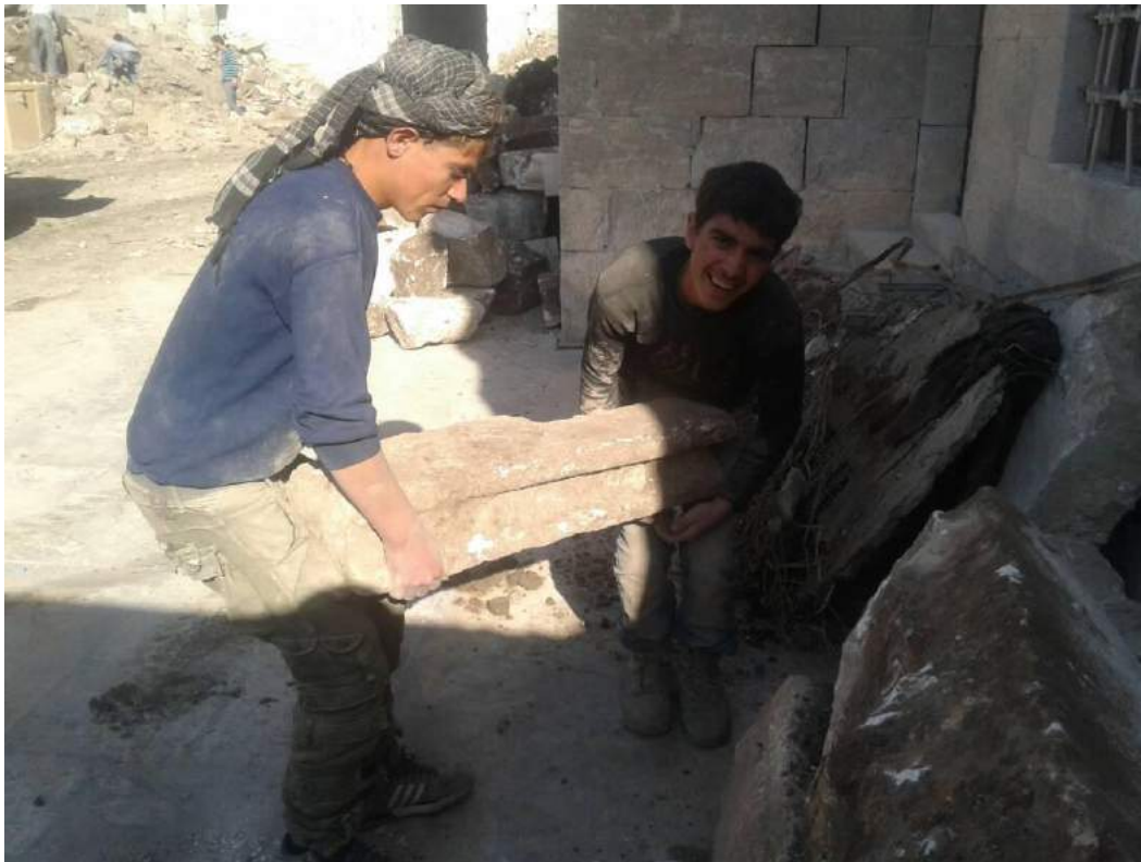
Workers sort rubble in the damaged northwest corner of museum (TDA-HPI; January 6, 2018)
