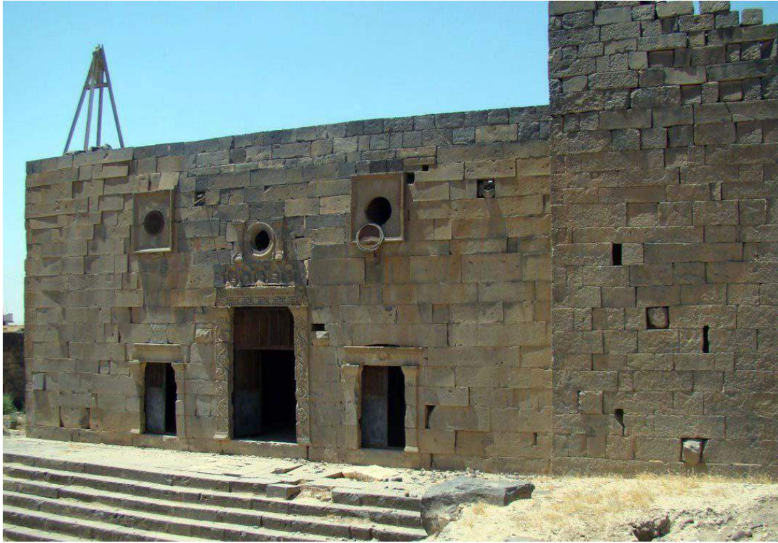
Facade of al-Mataiya Temple after repairs to stairs and roof above leftmost window (Al-Hkeka; January 23, 2018)
