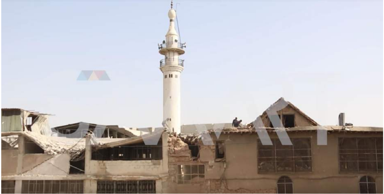
Video still of damage to exterior of al-Kabir Mosque (SMART News Agency; January 23, 2018)
