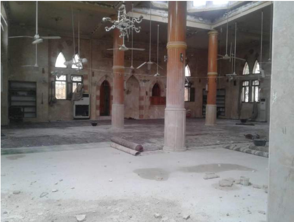
Damage to the interior of Uwais al-Qarni Mosque (ASOR CHI Source; January 4, 2018)
