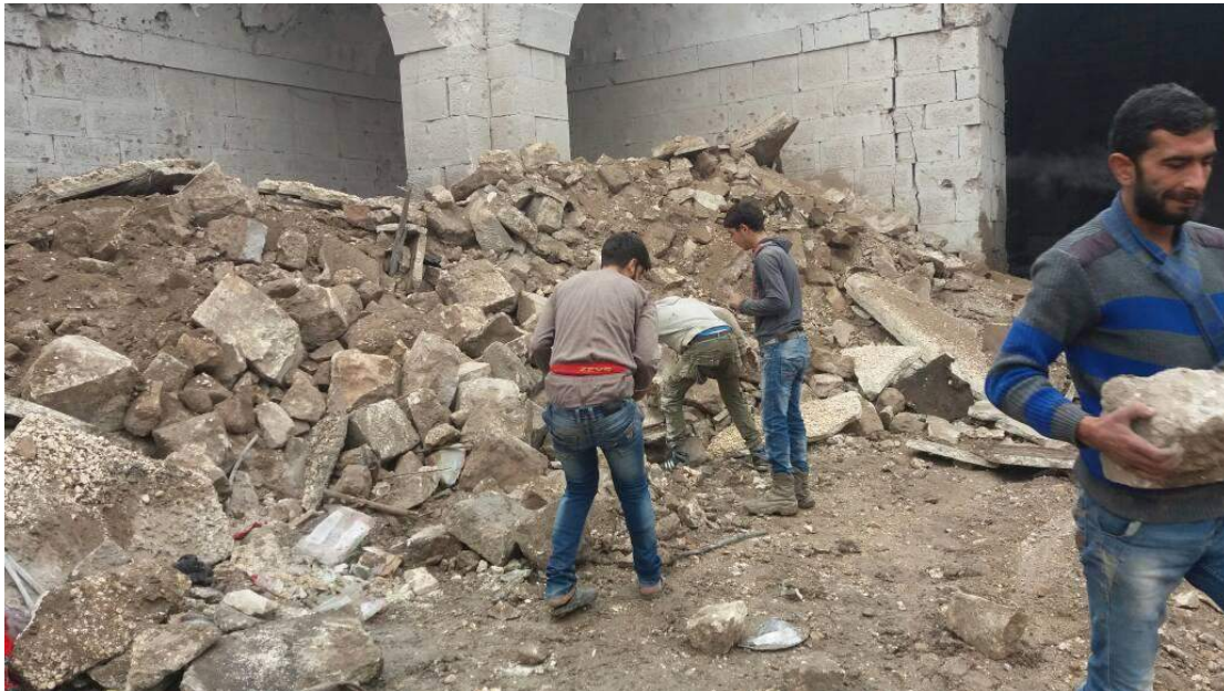
Workers sort through the rubble and collect fallen masonry in the damaged northwest corner (TDA-HPI; January 6, 2018)
