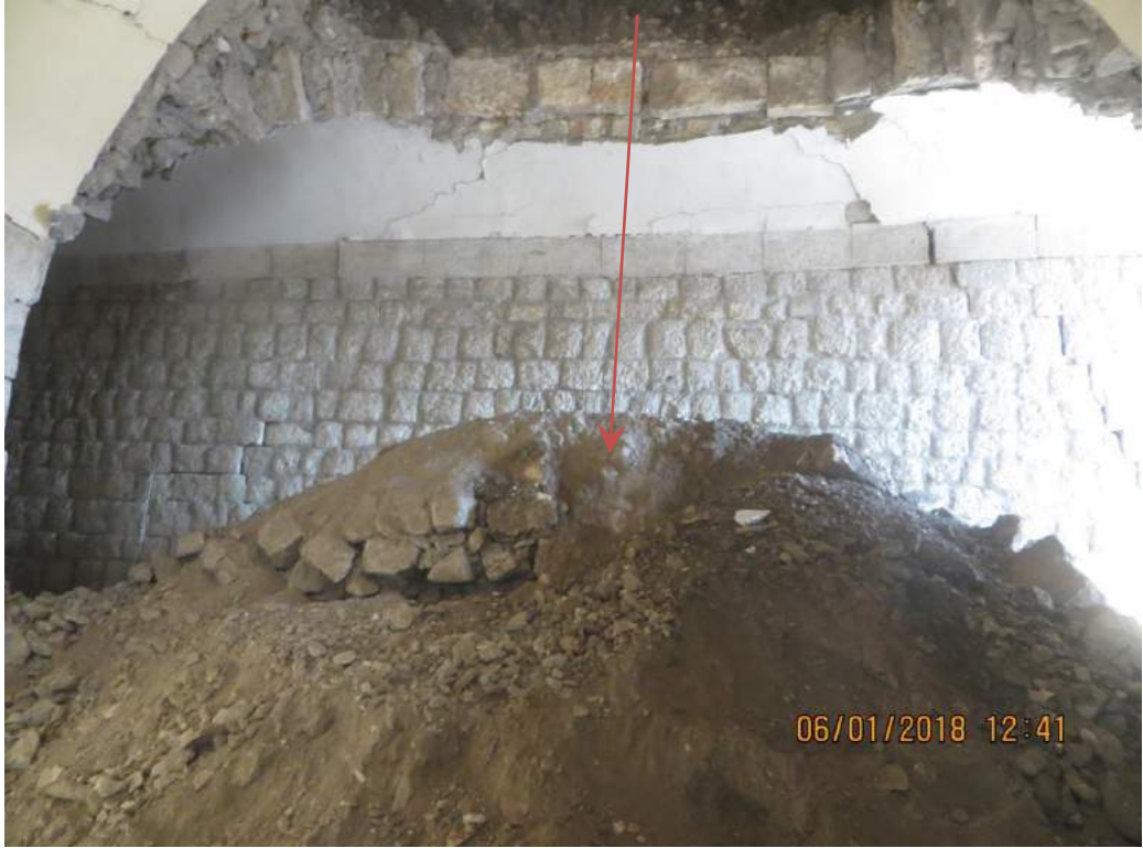
Rubble from collapsed roof rubble prior to commencement of work (TDA-HPI; January 6, 2018)
