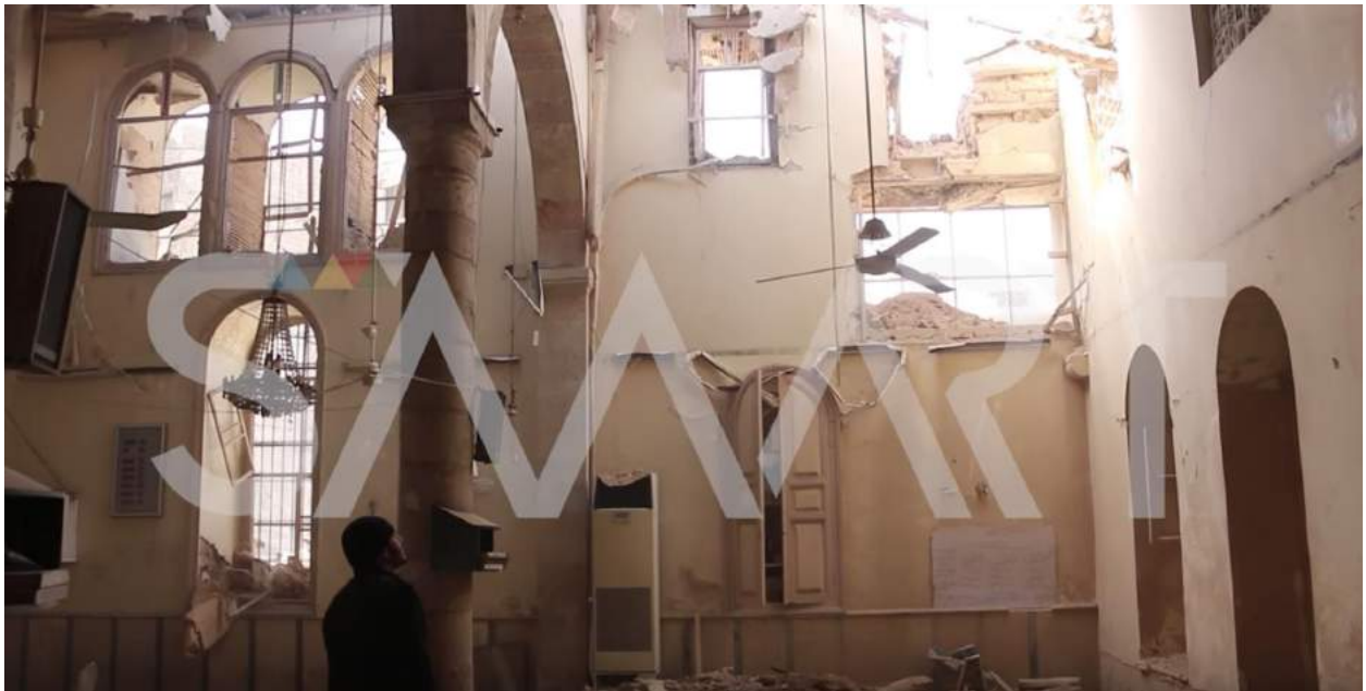
Video still of damage to interior of al-Kabir Mosque (SMART News Agency; January 23, 2018)
