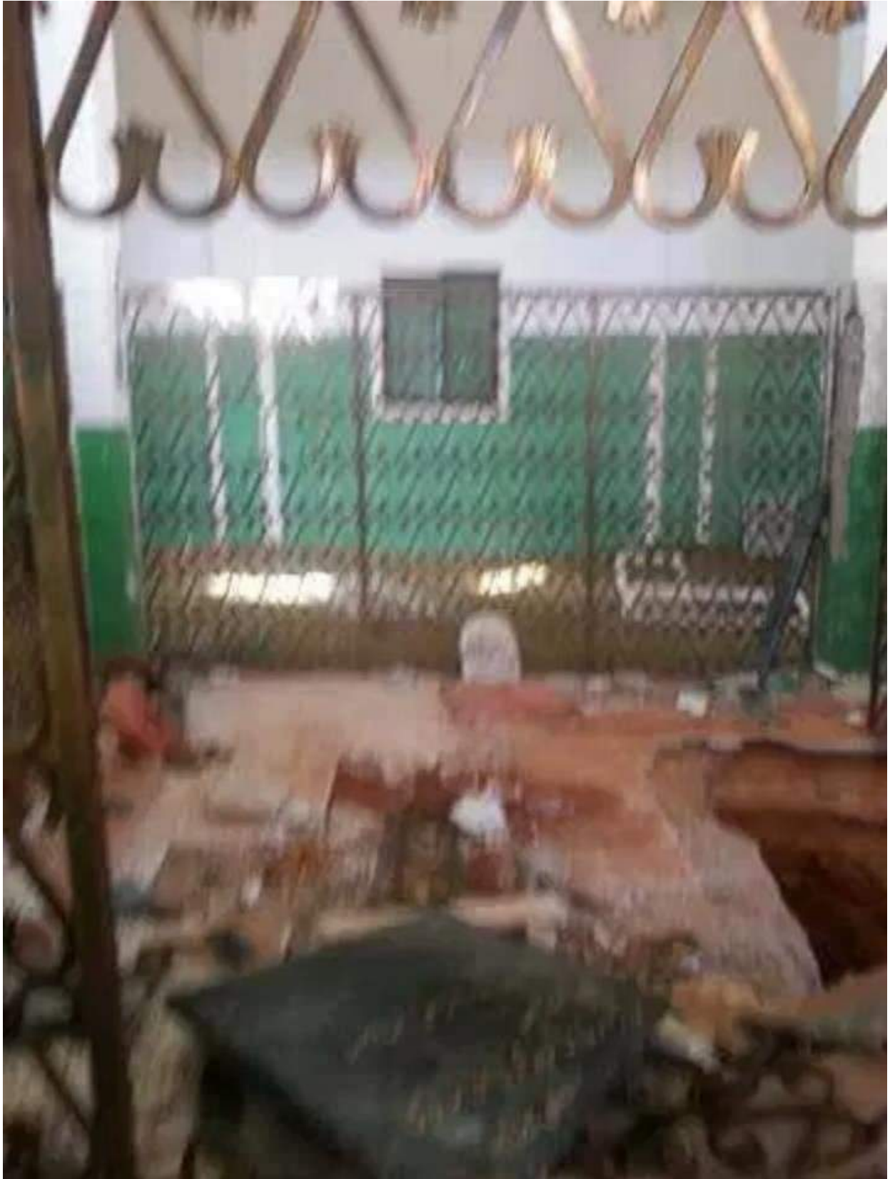
A view of the damage to the interior of the Mausoleum of al-Mahdi (Al Marsad; December 30, 2017)
