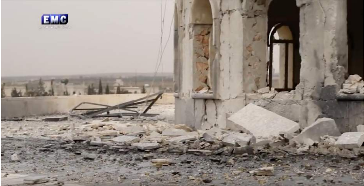
Video still of damage to the dome of al-Kabir Mosque (Edlib Media Center; January 4, 2018)
