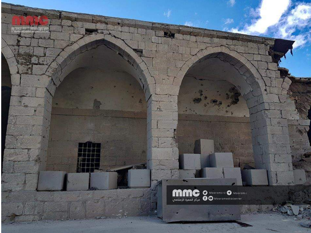
Damage to western arcade in interior courtyard of al-Ma'arra Museum (Maara Media Center/Twitter; January 2, 2018)
