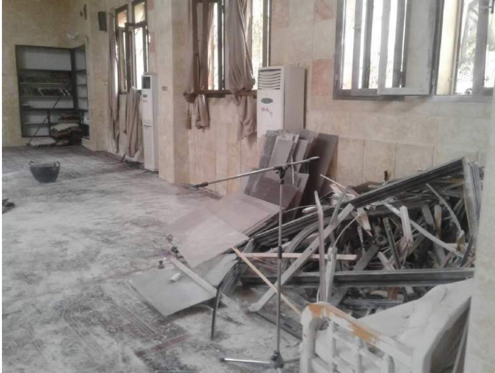
Damage to the interior of Uwais al-Qarni Mosque (ASOR CHI Source; January 4, 2018)
