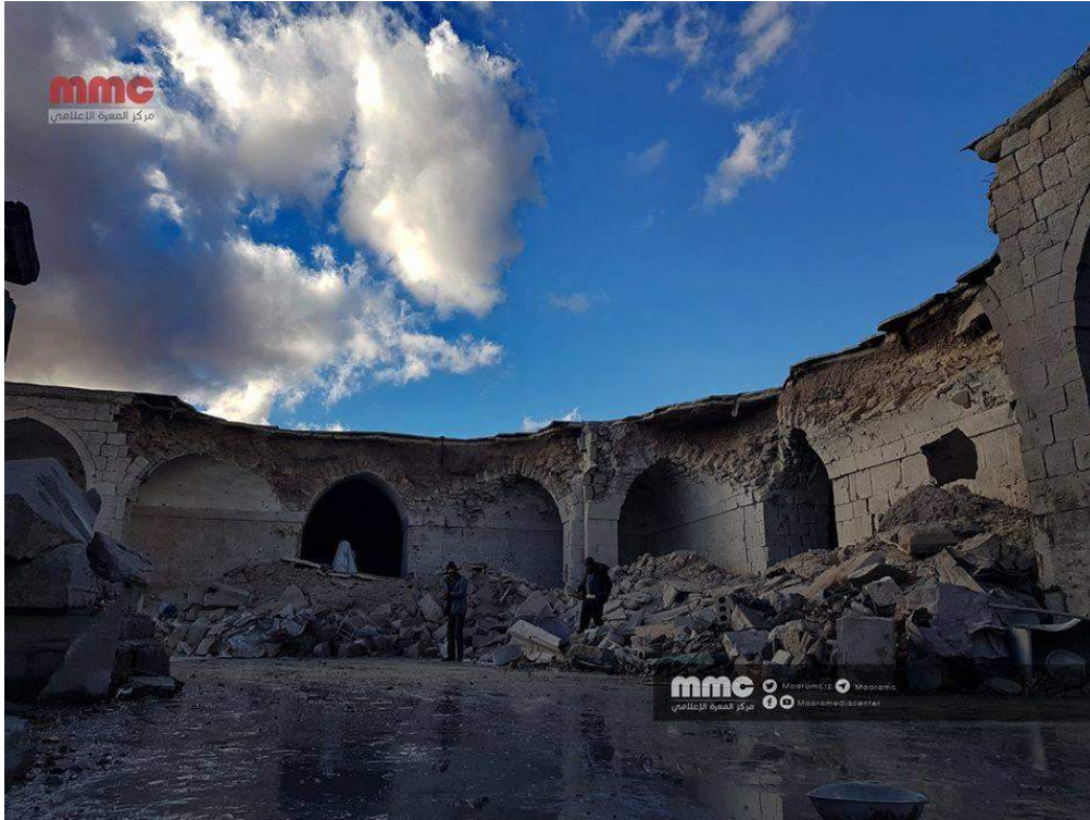
Damage to northeastern corner of courtyard arcade of al-Ma'arra Museum (Maara Media Center/Twitter; January 2, 2018)
