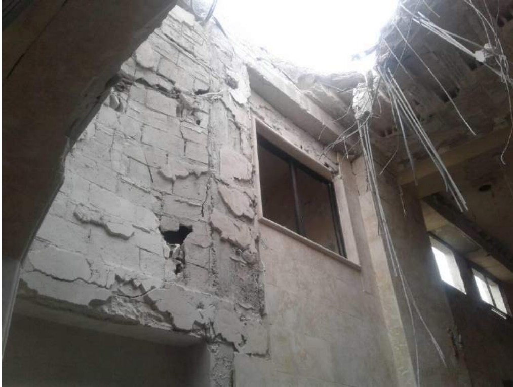
Damage to the interior of Uwais al-Qarni Mosque (ASOR CHI Source; January 4, 2018)
