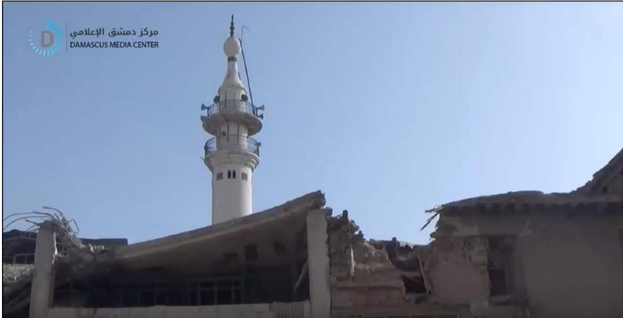
Video still of damage to al-Rahman Mosque exterior (Damascus Media Center; January 22, 2018)
