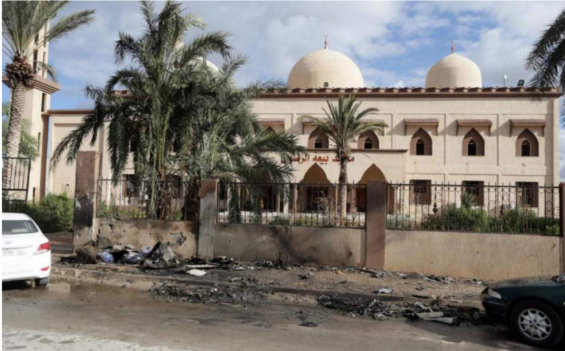
Damage to the wall around the Bayaat al-Radwan Mosque complex (Reuters; January 24, 2018)
