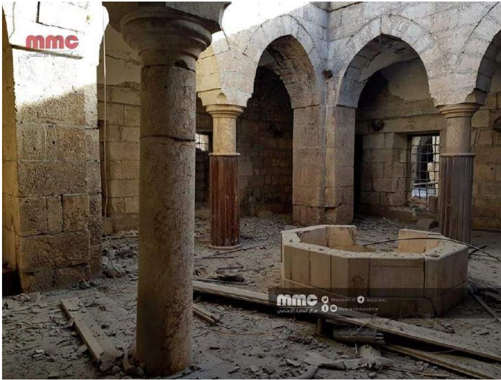
Damage to interior of tekkiye within interior courtyard of al-Ma'arra Museum (Maara Media Center/Twitter; January 2, 2018)
