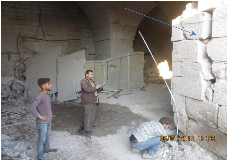
Workers assess damage to interior hallways of northwest corner of museum (TDA-HPI; January 6, 2018)
