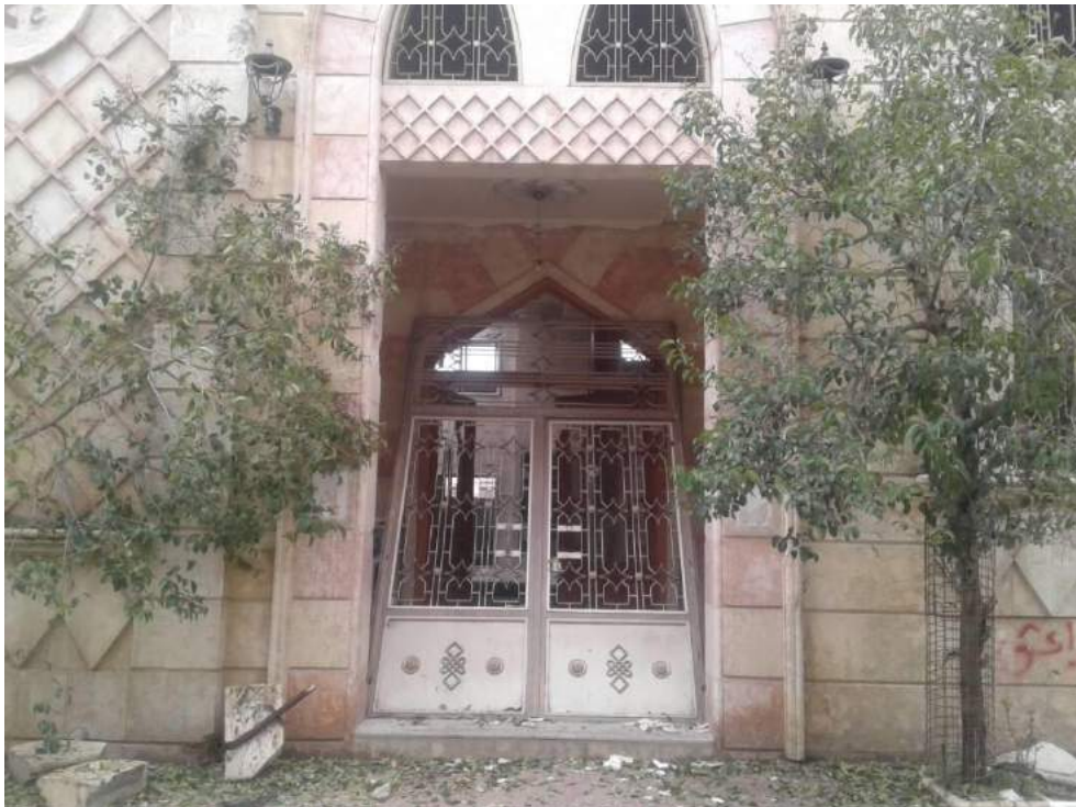
Damage to the exterior of Uwais al-Qarni Mosque (ASOR CHI Source; January 4, 2018)
