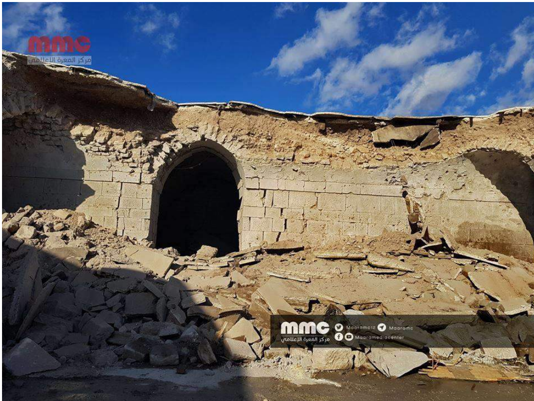
Damage to northern arcade of al-Ma'arra Museum (Maara Media Center/Twitter; January 2, 2018)
