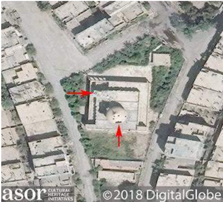
Damage to the minaret and the dome of Othman Bin Affan Mosque, indicated with red arrows (DigitalGlobe NextView License; September 16, 2014)
