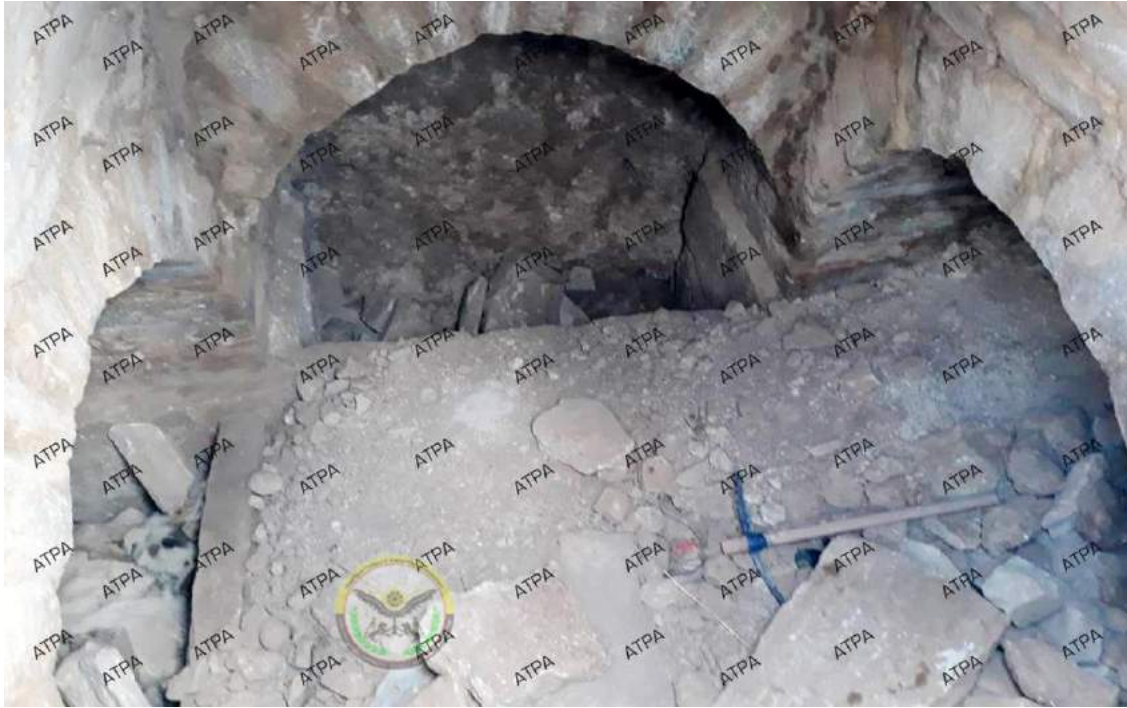
Interior of al-Farahia Byzantine tomb with debris from illegal excavation (ATPA; January 4, 2018)
