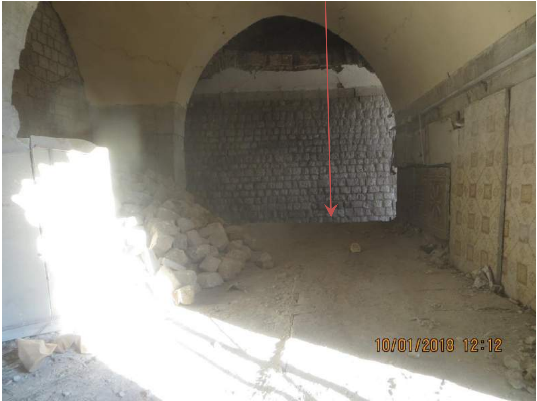
Area where roof collapsed removal of rubble (TDA-HPI; January 10, 2018)
