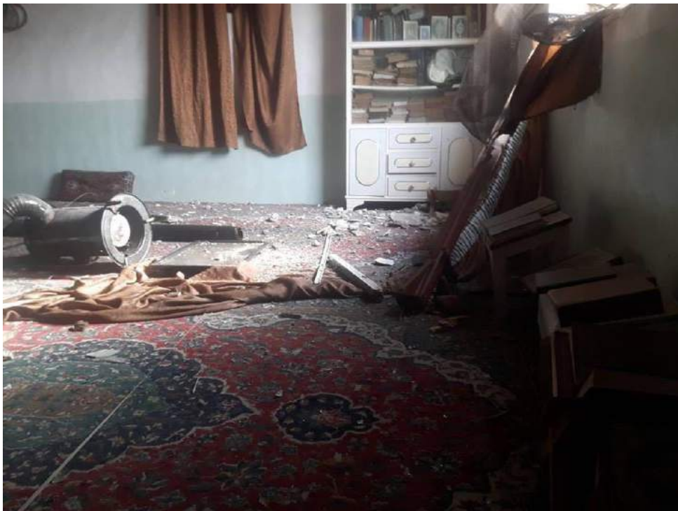
Damage to the interior of Salah al-Din al-Ayoubi Mosque (SOHR; January 27, 2018)
