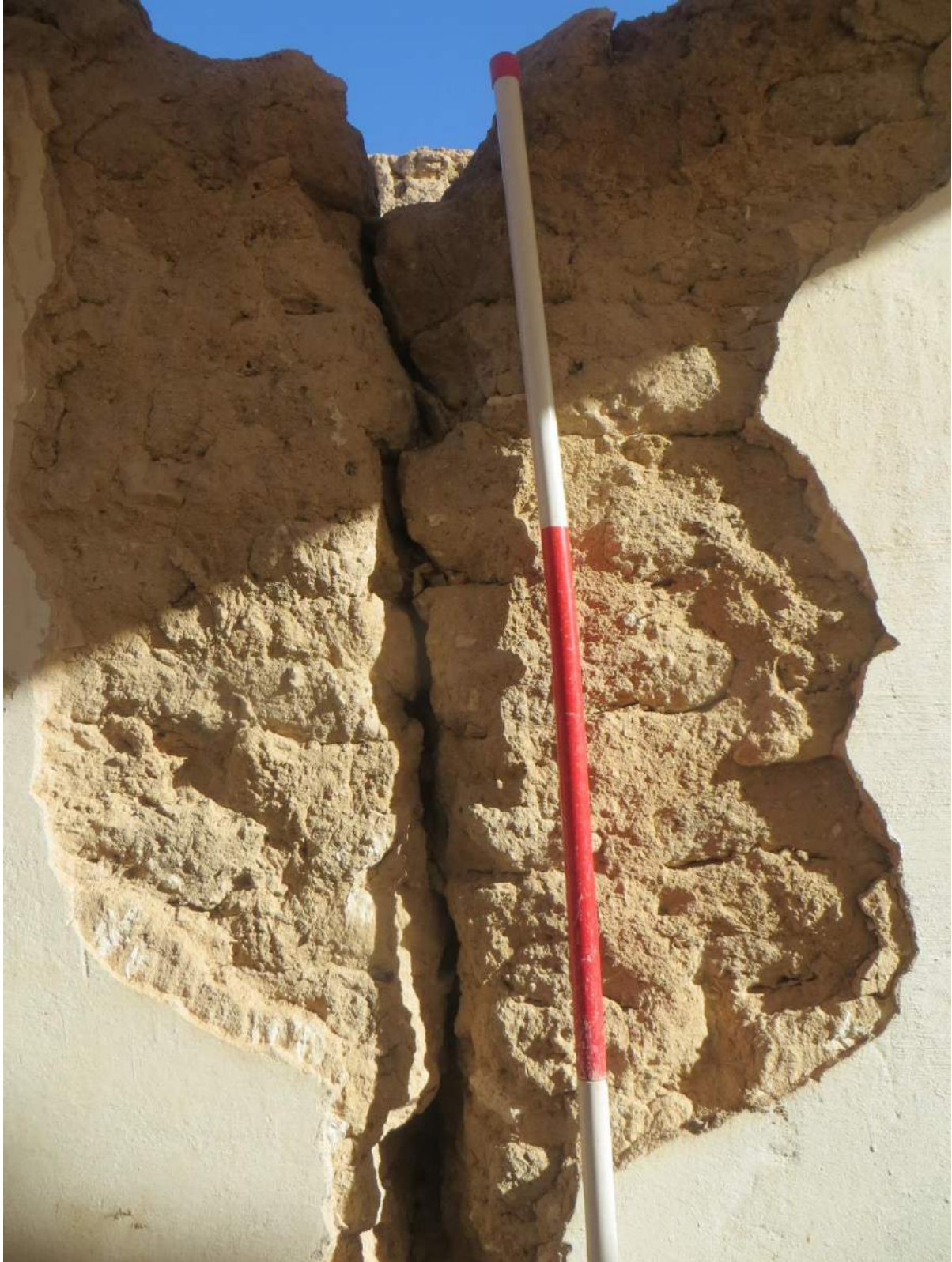
Plaster coatings that commonly protect the buildings in Ghadames have not been maintained, allowing cracks to propagate quickly during a rain storm (Mahmoud Hadia, December 27, 2017)
