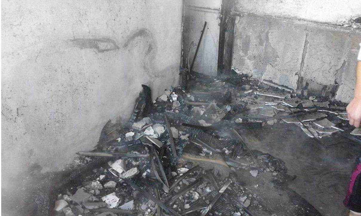
Fire damage in interior of Kaab bin Malik Mosque (Al-Zahra Neighborhood News Network; January 29, 2018)
