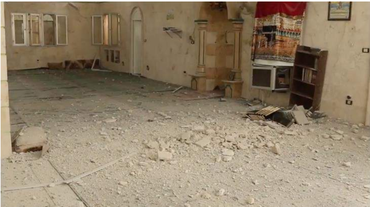
Video still of damage to the interior of al-Huda Mosque (Edlib Media Center; January 21, 2018)
