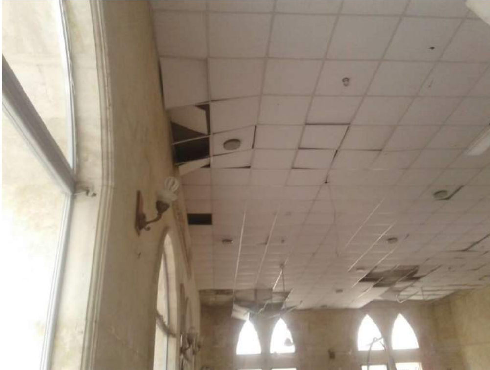
Damage to the interior of Uwais al-Qarni Mosque (ASOR CHI Source; January 4, 2018)
