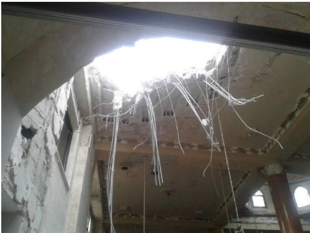
Damage to the interior of Uwais al-Qarni Mosque (ASOR CHI Source; January 4, 2018)
