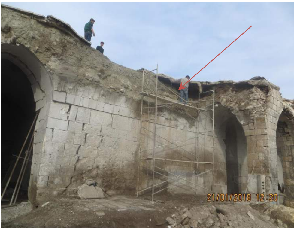
Workers filled cracks with 400 kg/m 3 grade cement. The surface of the cracks were then plastered over and treated with acrylic to prevent water seepage (TDA-HPI; January 21, 2018)
