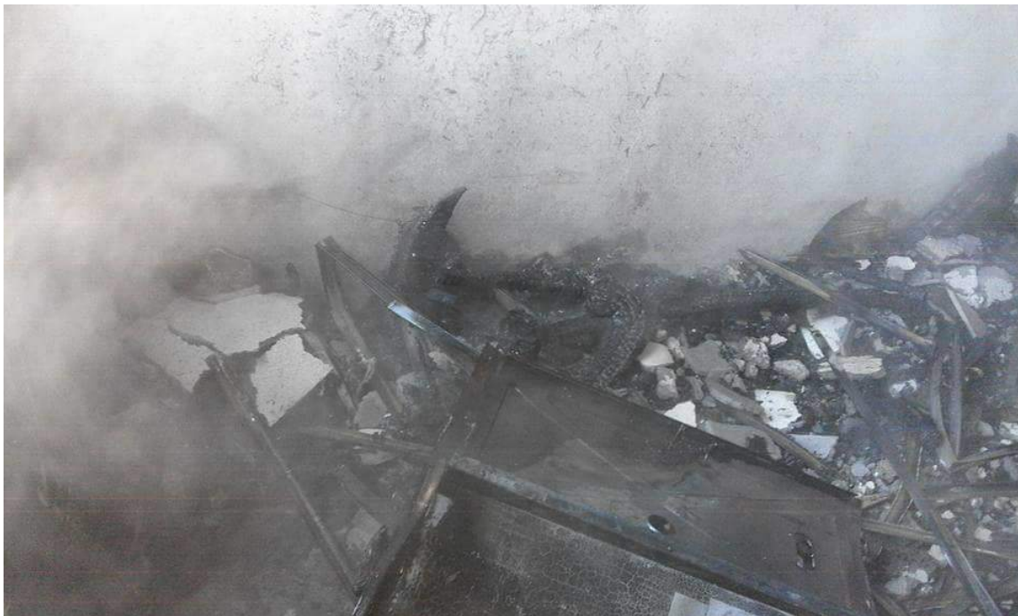
Fire damage in interior of Kaab bin Malik Mosque (Al-Zahra Neighborhood News Network; January 29, 2018)
