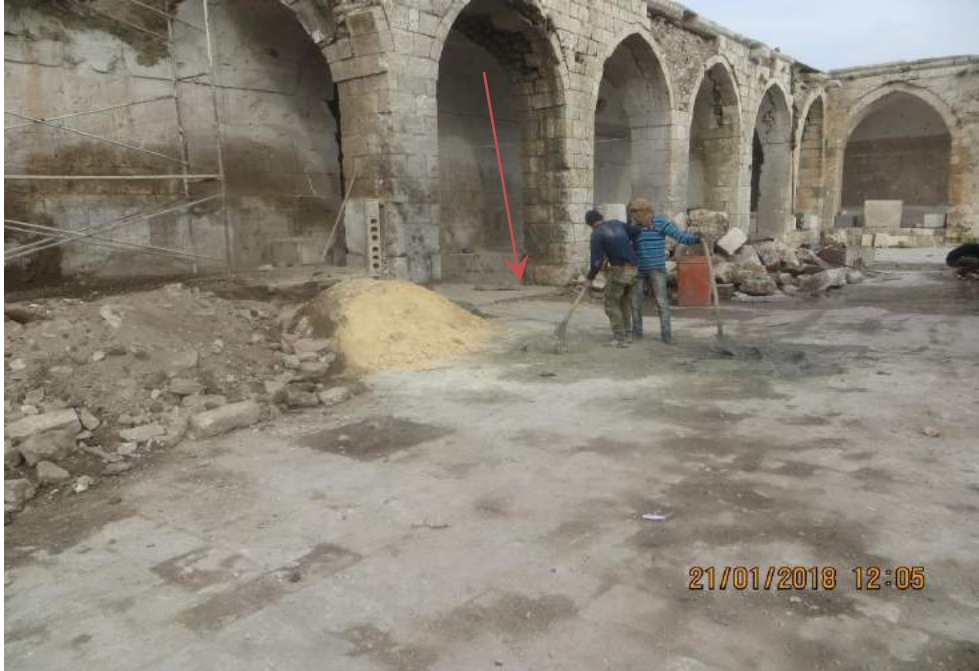
Workers prepare cement mix and apply it to damaged areas (TDA-HPI; January 21, 2018)
