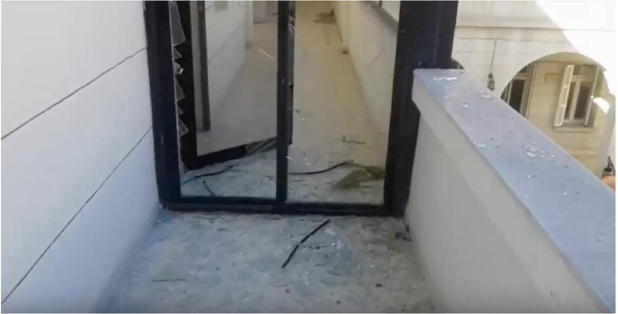
Damage to doors on second floor of Maronite Church (Dimashq Now; January 8, 2018)
