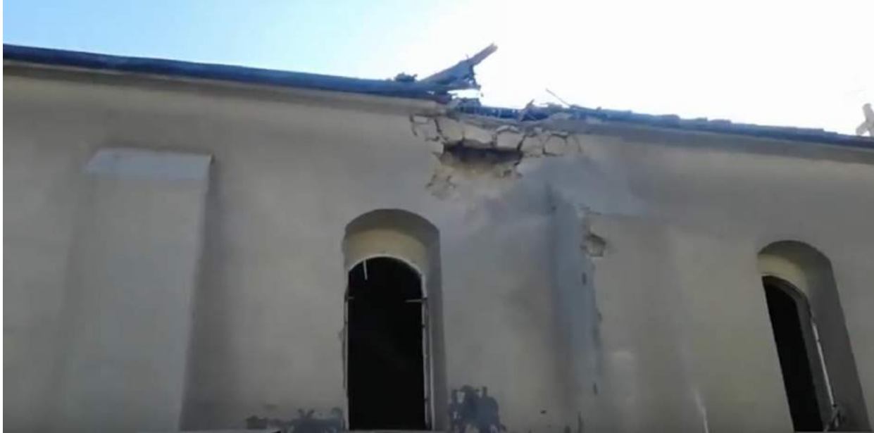
Damage to the roof of Latin Church (Dimashq Now; January 8, 2018)
