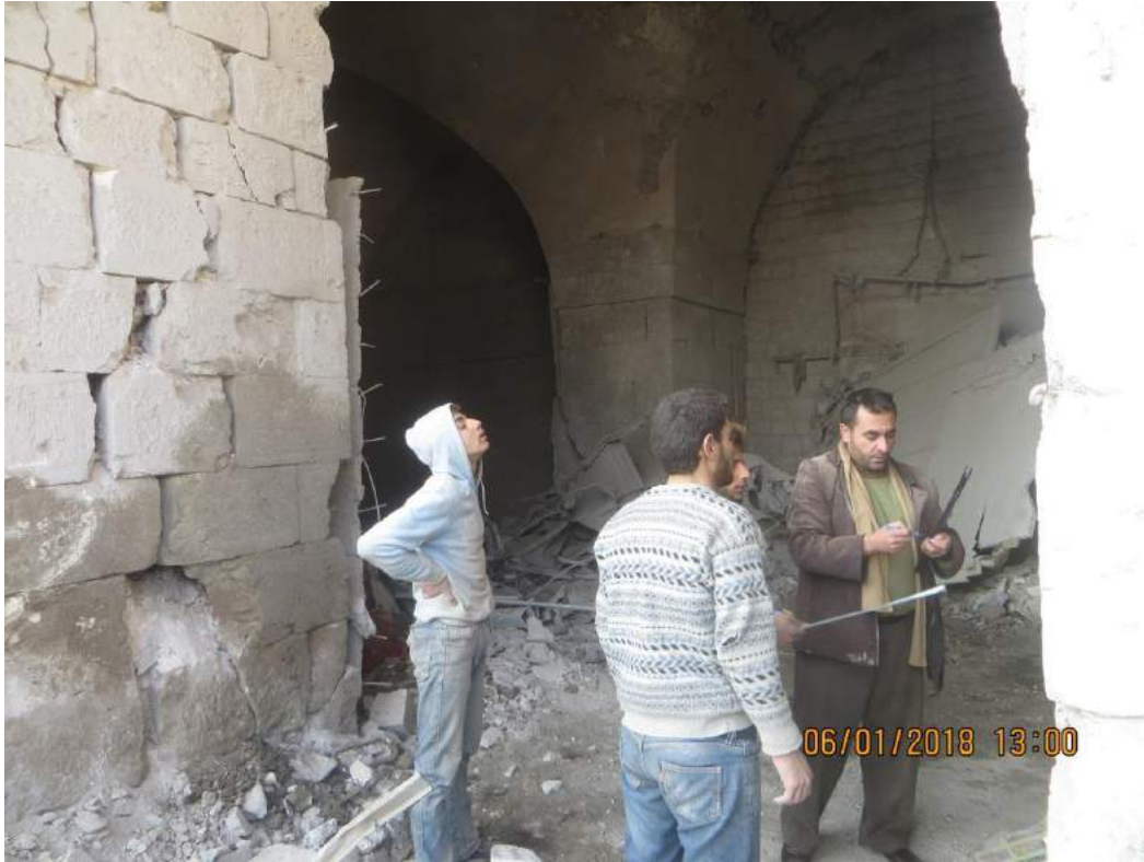
Workers assess damage and take measurements (TDA-HPI; January 6, 2018)
