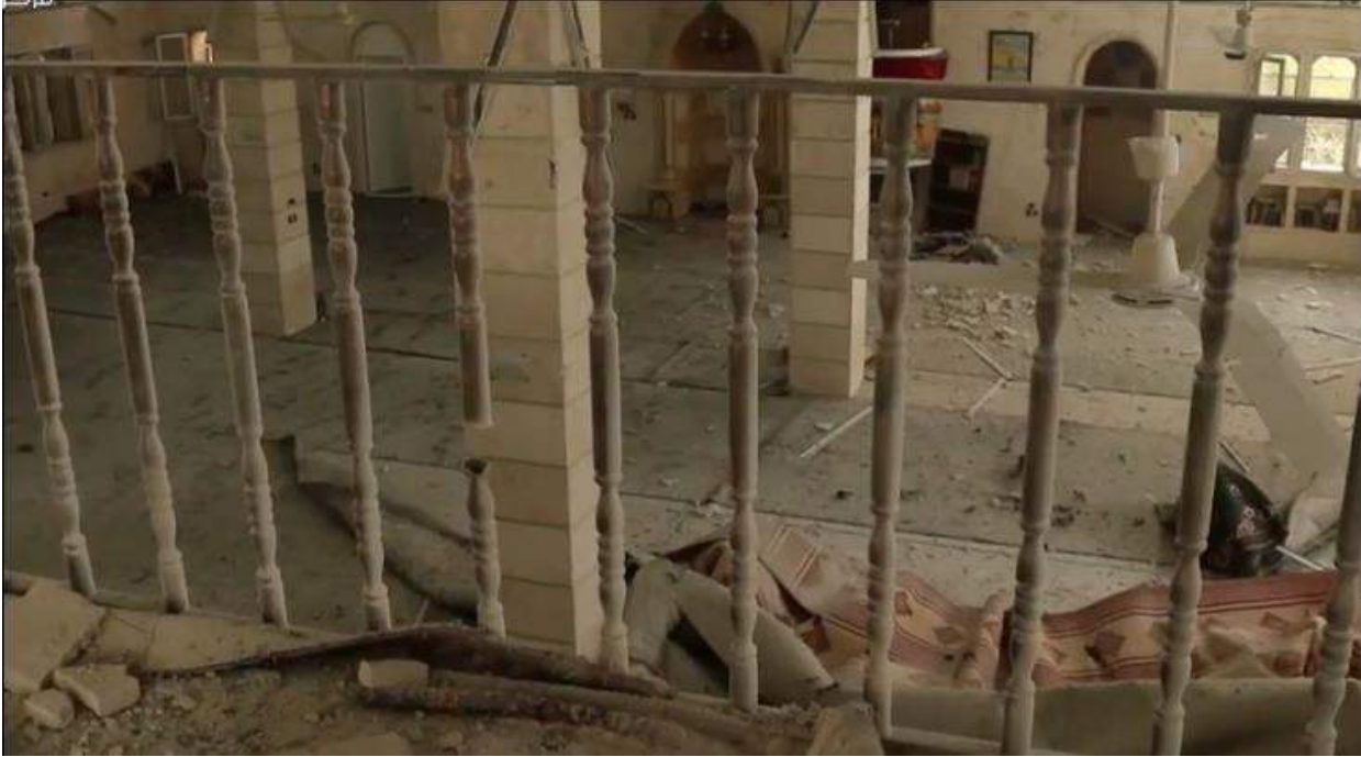
Video still of damage to the interior of al-Huda Mosque (Edlib Media Center; January 21, 2018)
