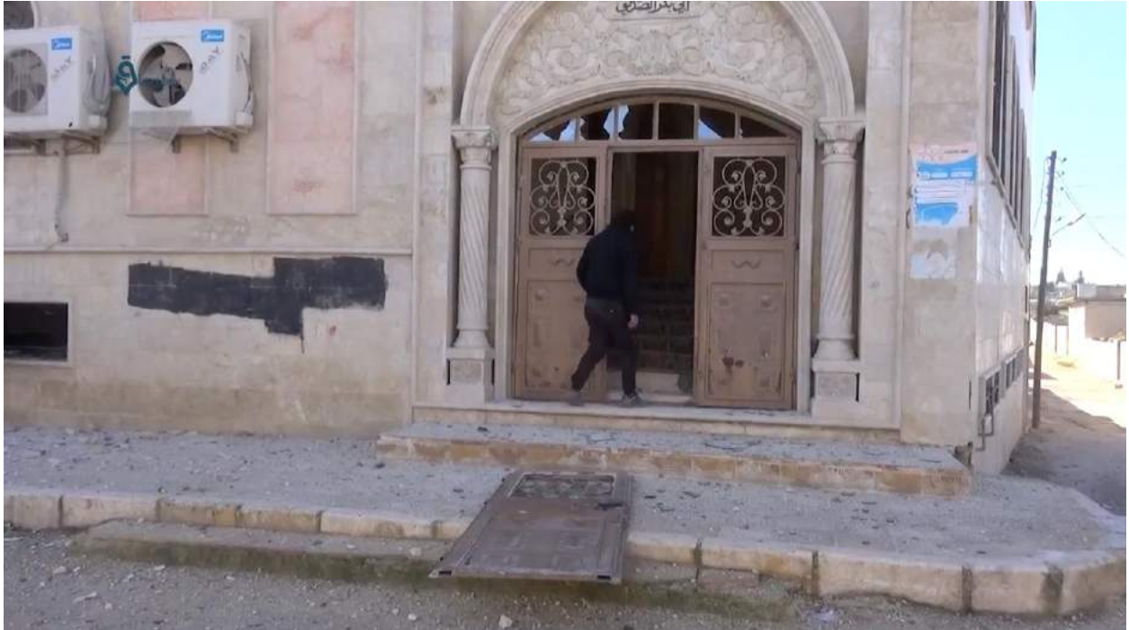
Video still of damage to exterior of Abu Bakr al-Siddiq Mosque (Qasioun News Agency; January 8, 2018)
