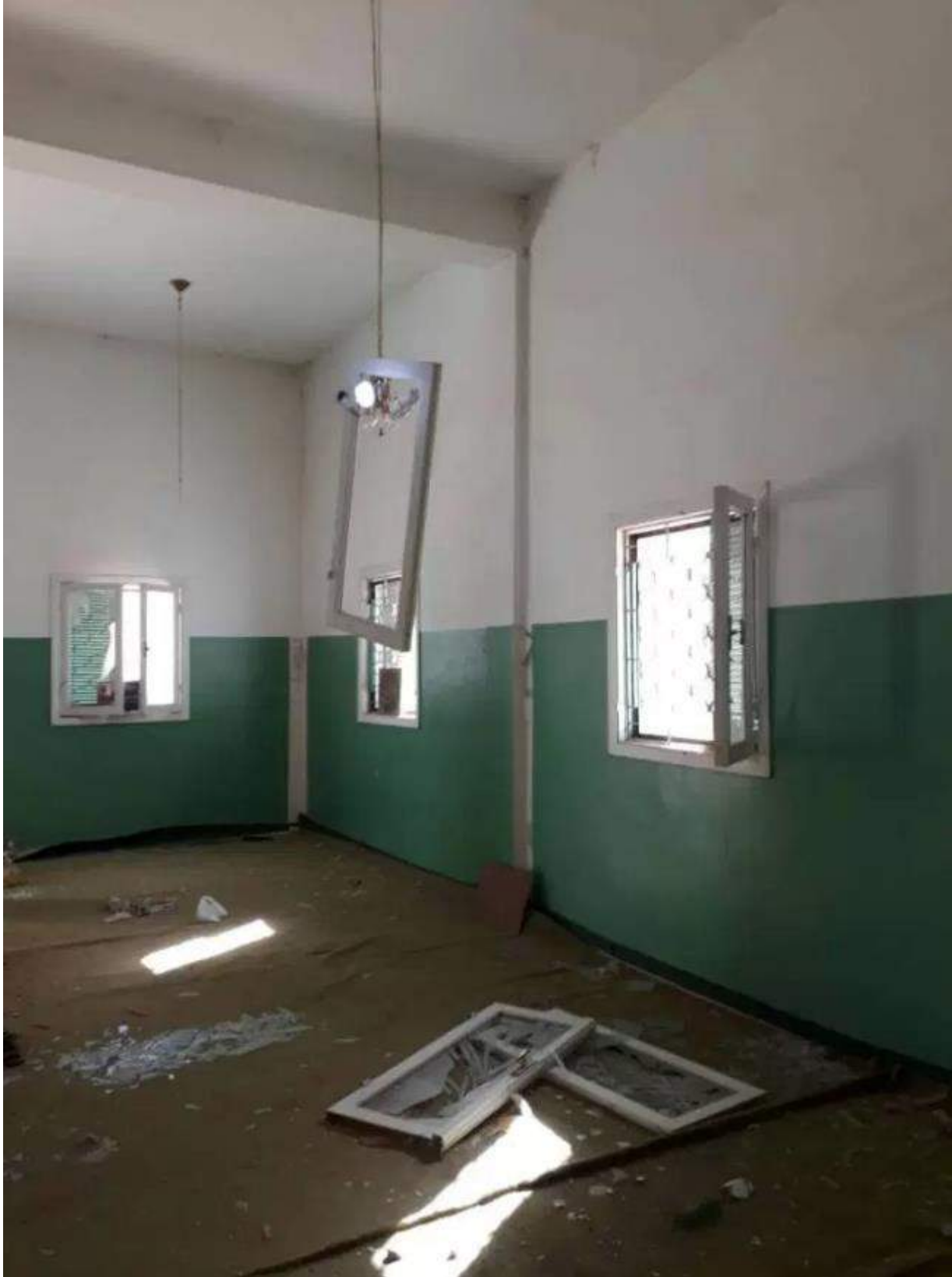
A view of the damage to the interior of the Mausoleum of al-Mahdi (Libyan Cloud News Agency; December 31, 2017)
