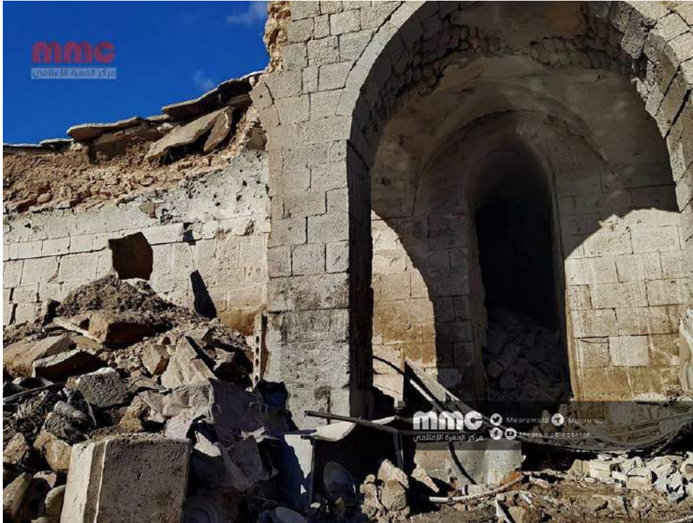
Damage to northern arcade of interior courtyard of al-Ma'arra Museum (Maara Media Center/Twitter; January 2, 2018)
