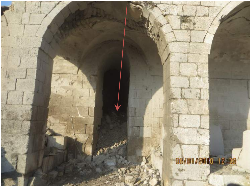
Gallery entrance before workers cleared rubble (TDA-HPI; January 6, 2018)
