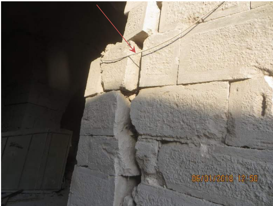
Image of damaged masonry blocks (TDA-HPI; January 6, 2018)
