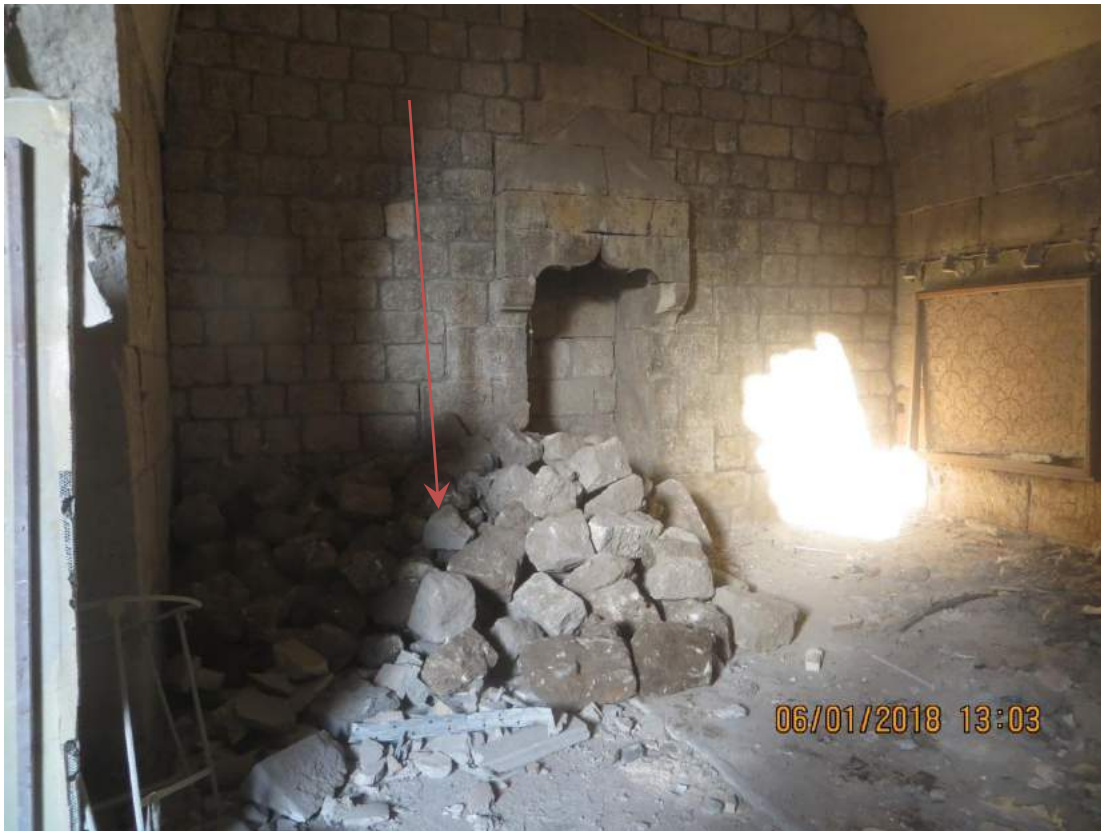
Workers gathered collapsed masonry (TDA-HPI; January 6, 2018)
