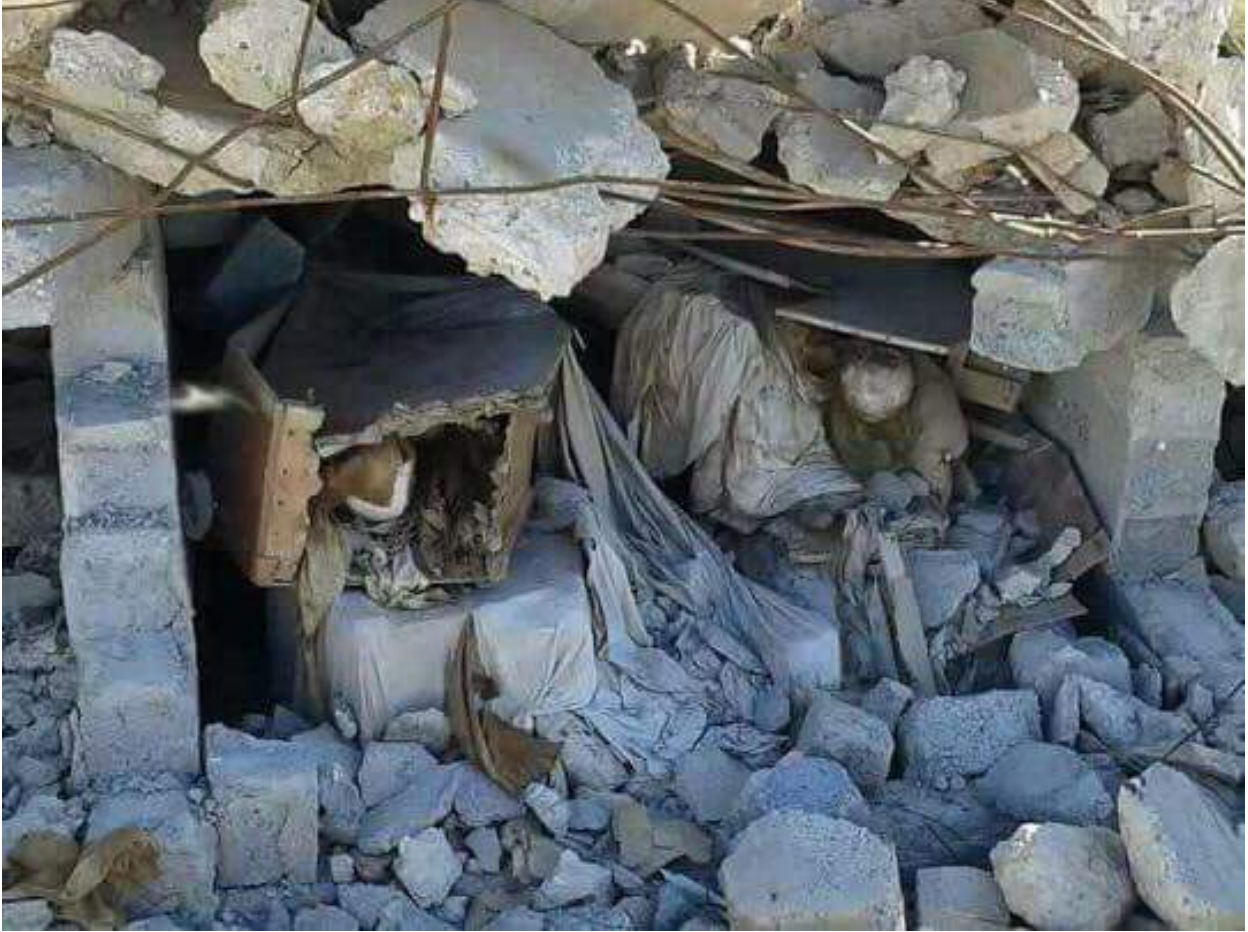
Damaged tombs and remains at Wadi 'Ikab Cemetery (This is Christian Iraq/Facebook; January 16, 2018)
