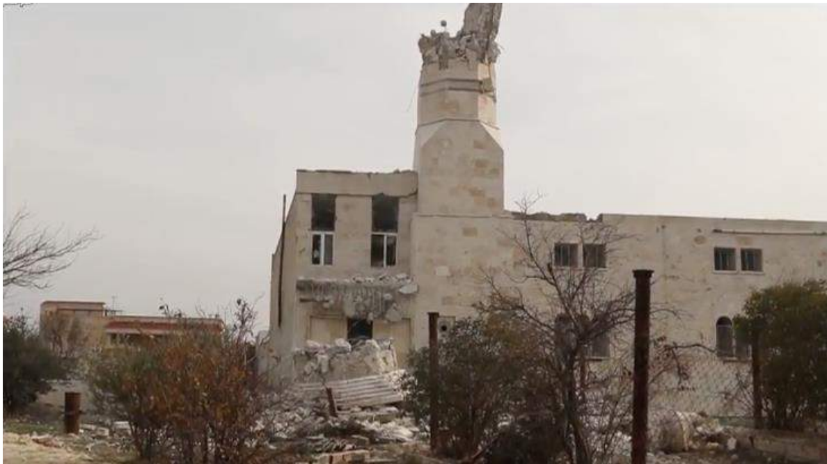
Video still of the destroyed minaret and damage to al-Huda Mosque (Edlib Media Center; January 21, 2018)
