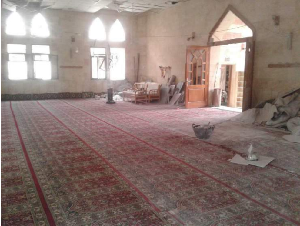
Damage to the interior of Uwais al-Qarni Mosque (ASOR CHI Source; January 4, 2018)
