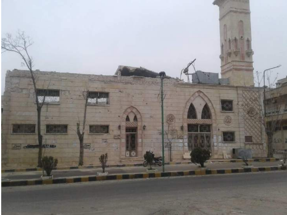
Damage to the exterior of Uwais al-Qarni Mosque (ASOR CHI Source; January 4, 2018)
