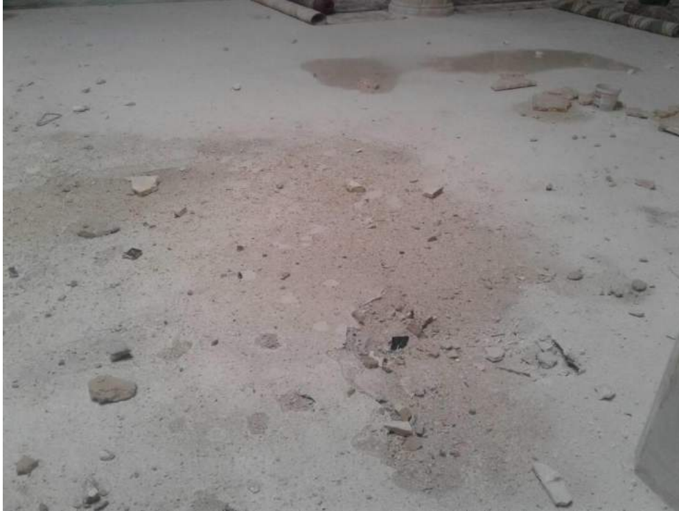
Damage to the interior of Uwais al-Qarni Mosque (ASOR CHI Source; January 4, 2018)
