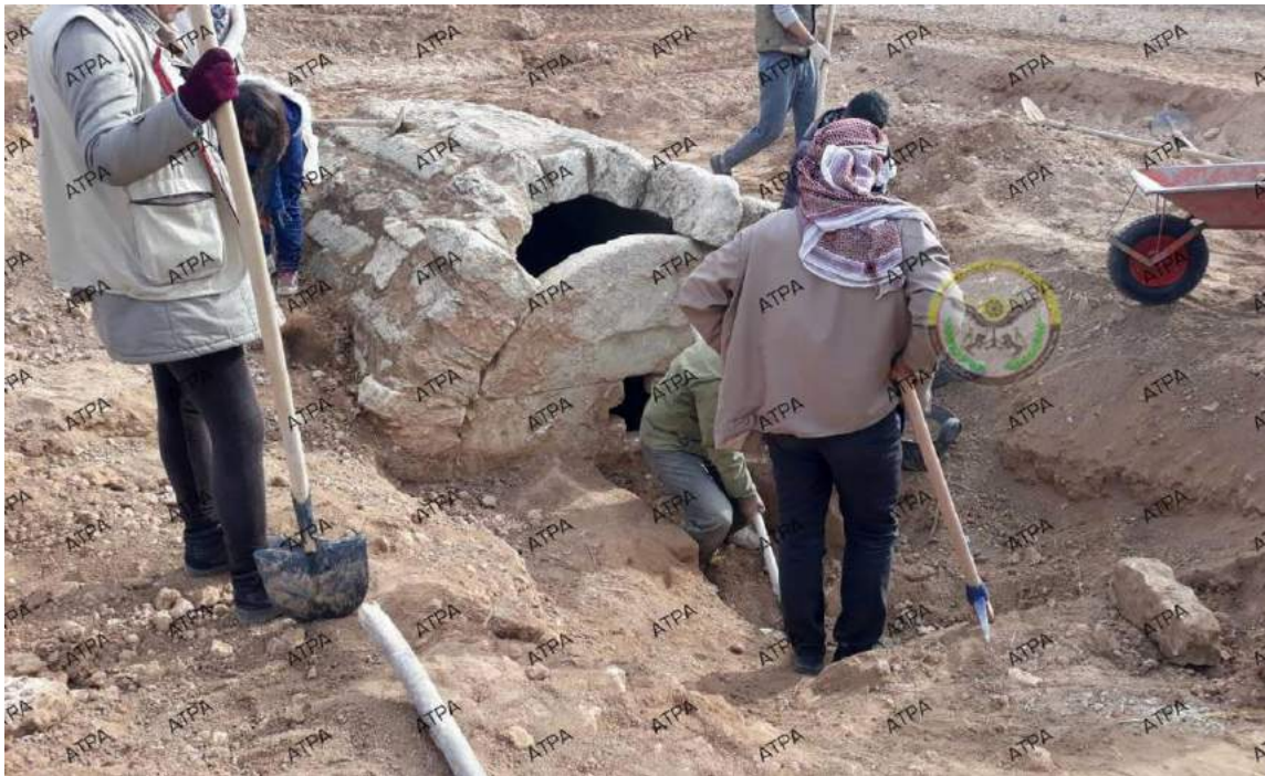
The ATPA conducts excavation and restoration work at al-Farahia Byzantine tomb (ATPA; January 4, 2018)
