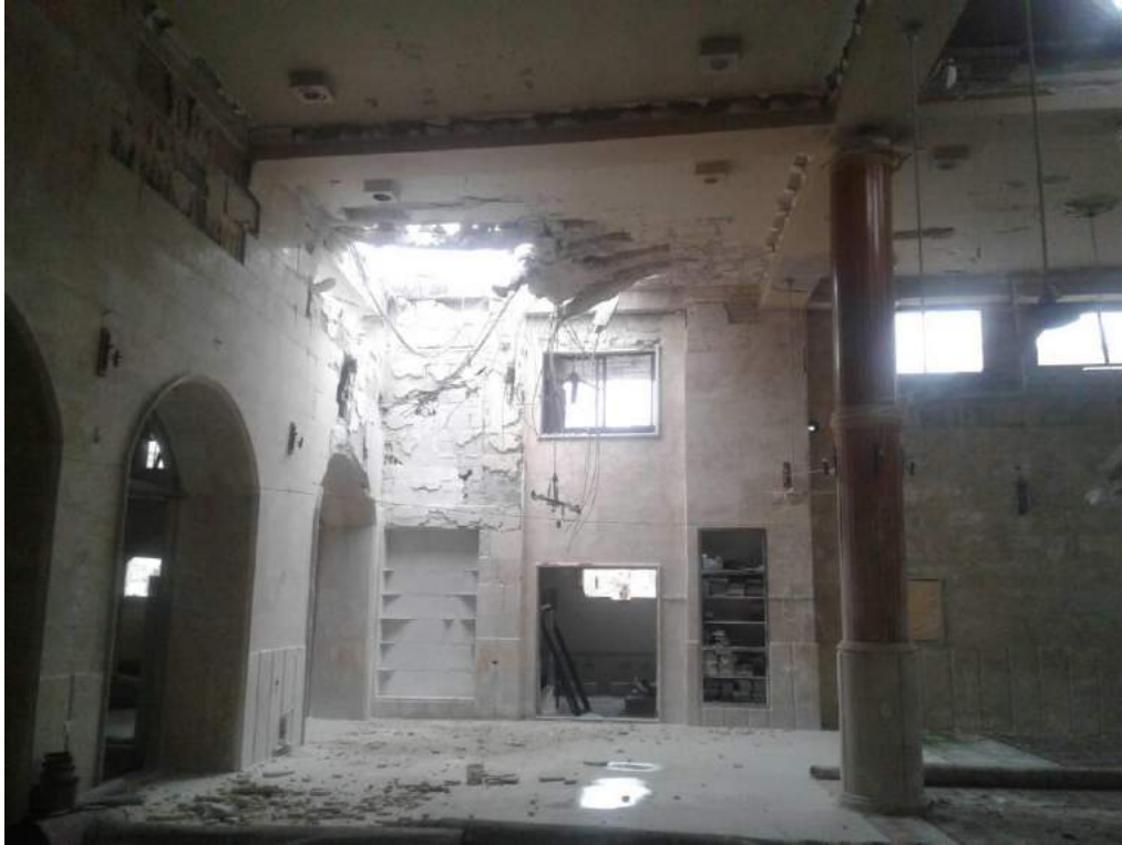
Damage to the interior of Uwais al-Qarni Mosque (ASOR CHI Source; January 4, 2018)
