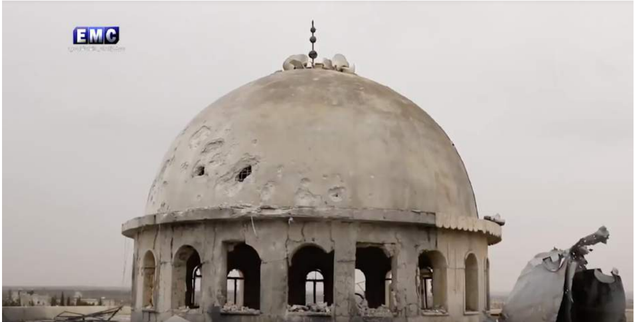
Video still of damage to the dome of al-Kabir Mosque (Edlib Media Center; January 4, 2018)
