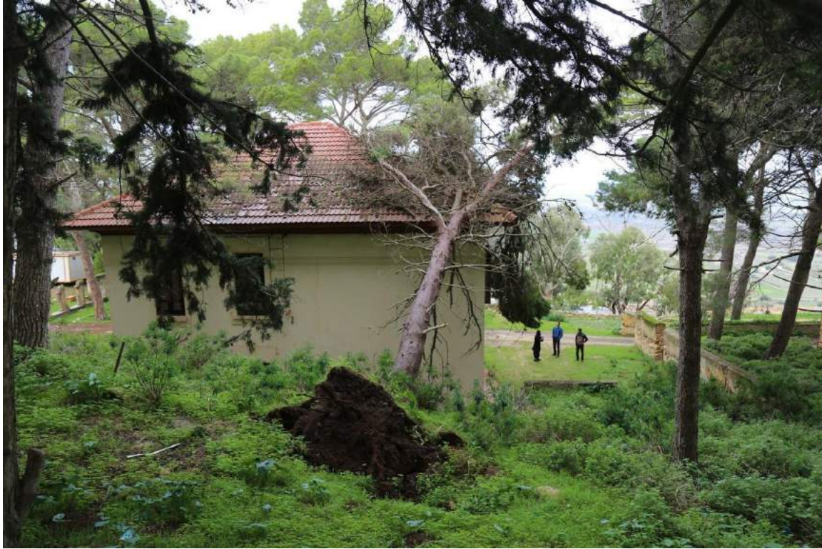
A view of the tree that fell on the roof of the DoA Shahat Library (DoA Shahat; January 4, 2018)
