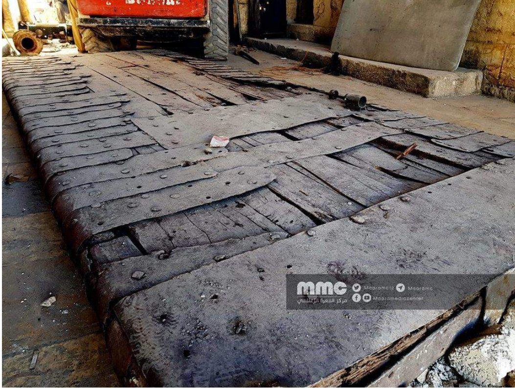
Damage to door in interior courtyard of al-Ma'arra Museum (Maara Media Center/Twitter; January 2, 2018)
