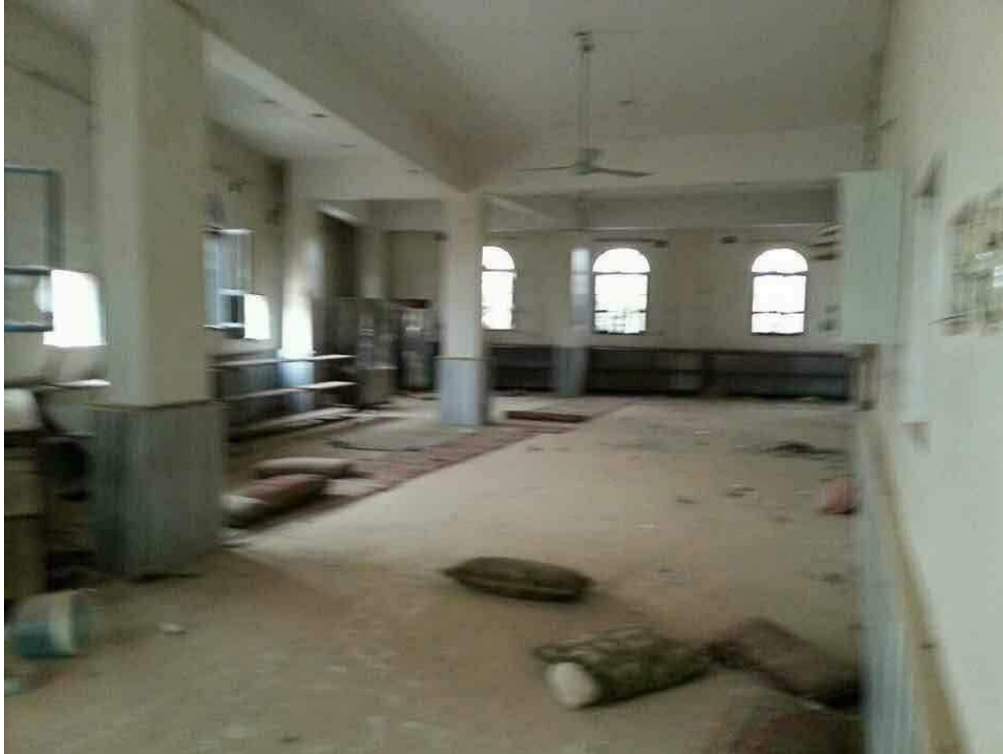
Damage to the interior of Khalid bin Walid Mosque (Euphrates Post; January 23, 2018)
