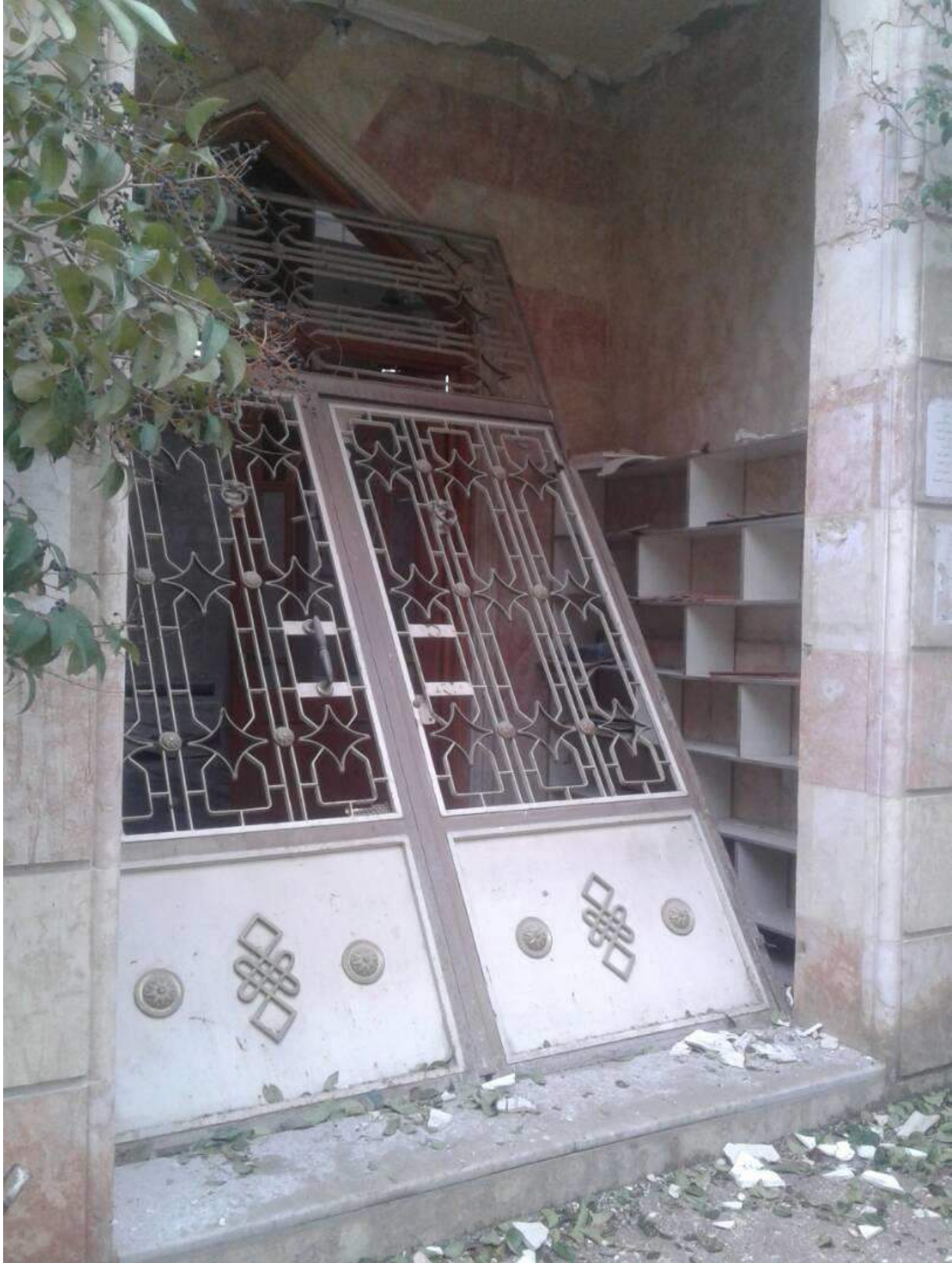
Damage to the exterior of Uwais al-Qarni Mosque (ASOR CHI Source; January 4, 2018)
