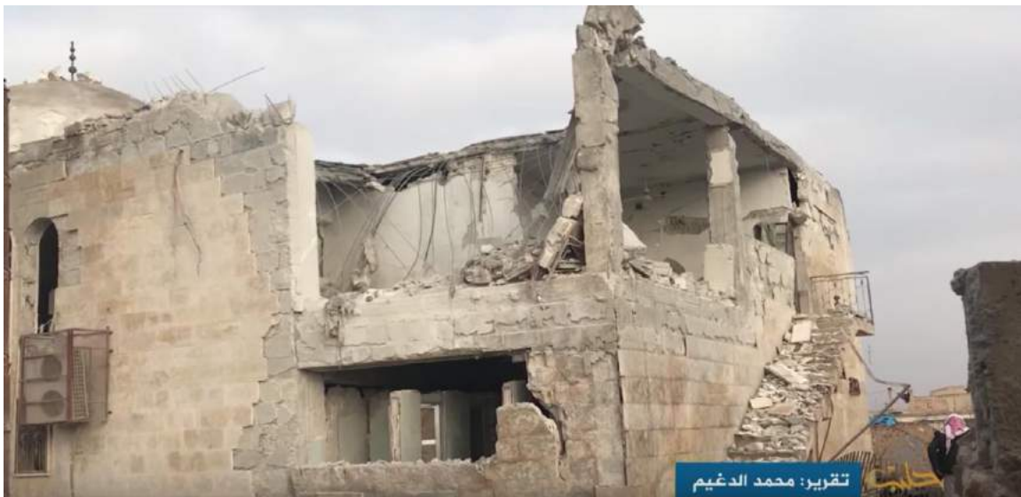
Video still of severe damage to the exterior of al-Kabir Mosque (Halab Today TV; January 4, 2018)
