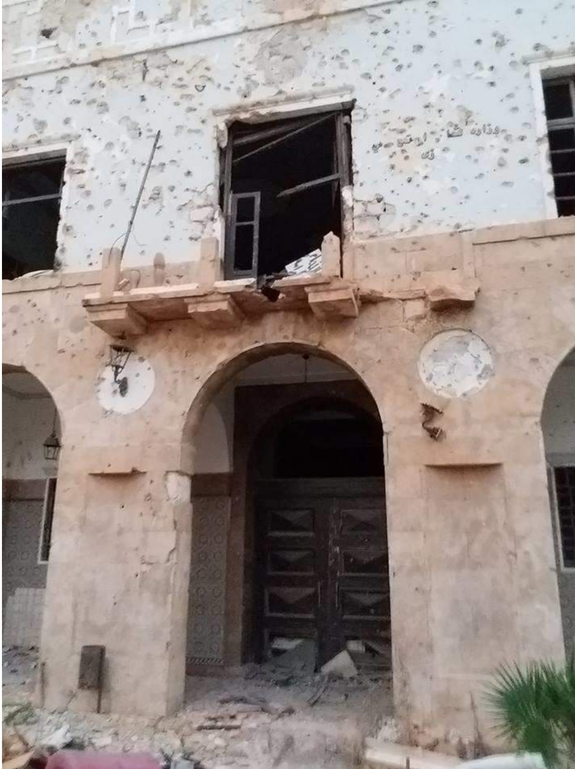
The current condition of the same balcony at Qasr al Manar (Private Facebook Account)
