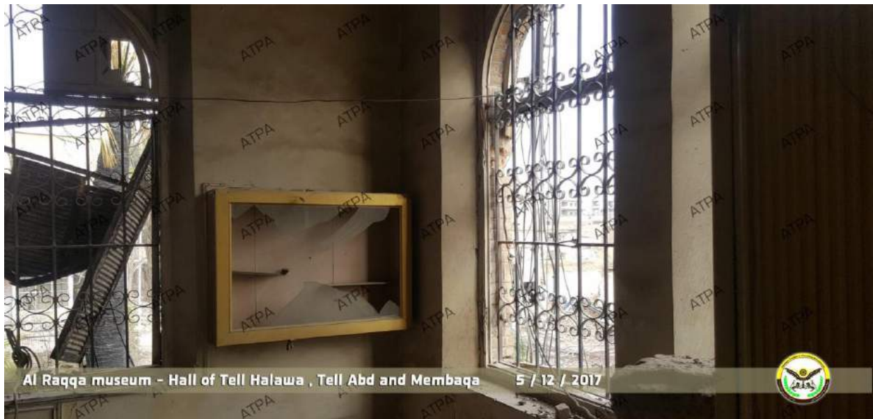
The exhibit room in the northeastern corner of the second floor, seen from the south (ATPA; December 11, 2017)
