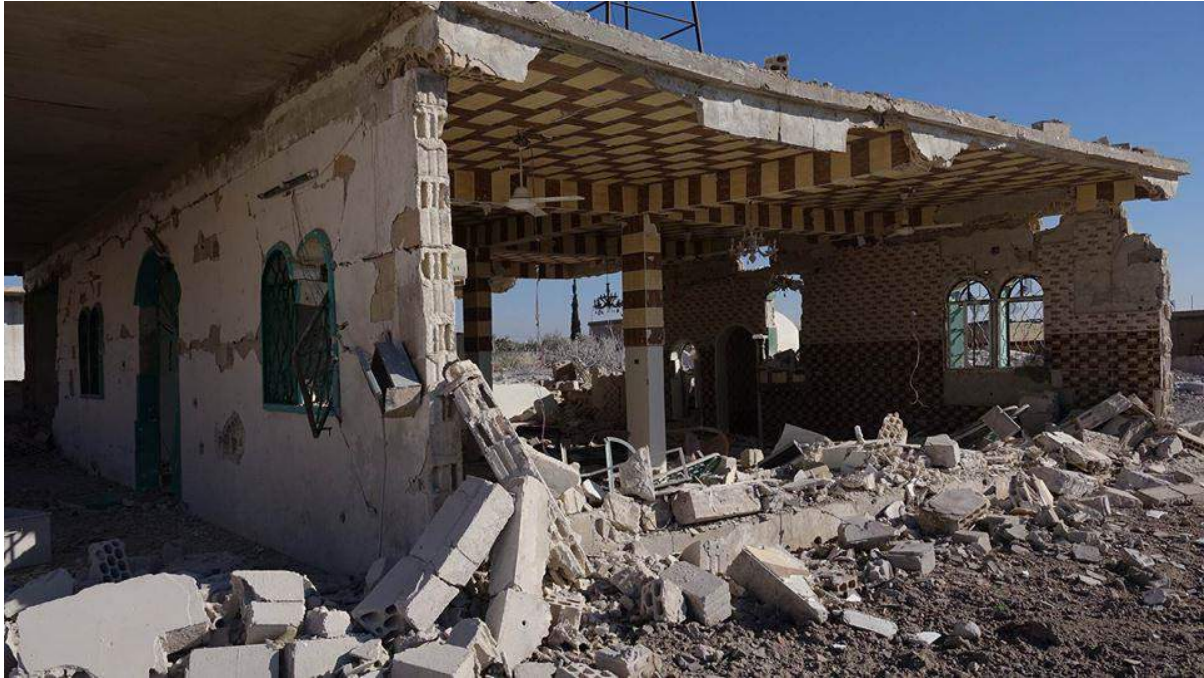
Partial destruction of mosque in the village of Zarzour (SNHR; December 9, 2017)
