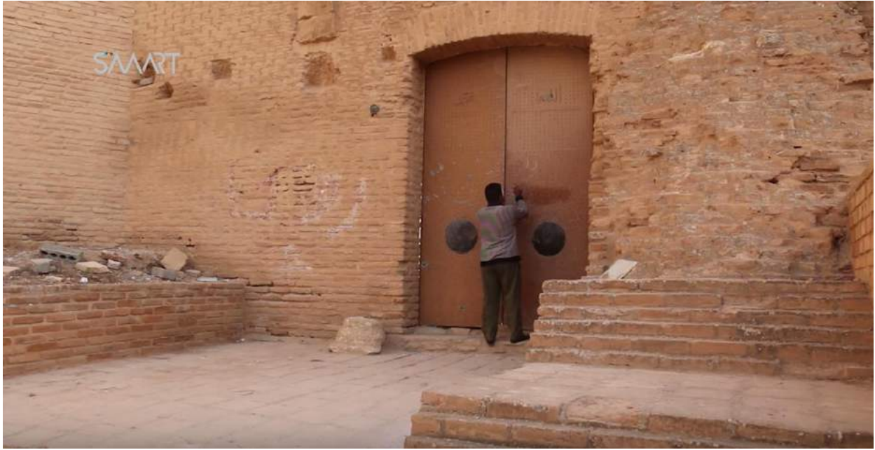
Graffiti on right side of the entrance has been cleaned up and the doors have been repaired (SMART News Agency; December 13, 2017)
