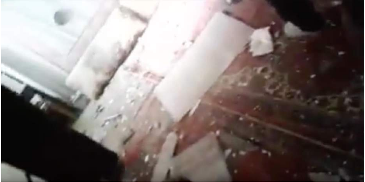
Video still of debris on the floor of al-Kabir Mosque, possibly from damaged ceiling tiles (SNHR; December 17, 2017)
