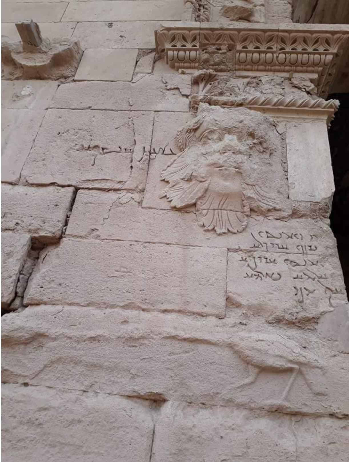
Intentional damage to gorgon image on left side of entrance to iwan on east side of side, as well as damage from weathering (ASOR CHI Source; December 14, 2017)
