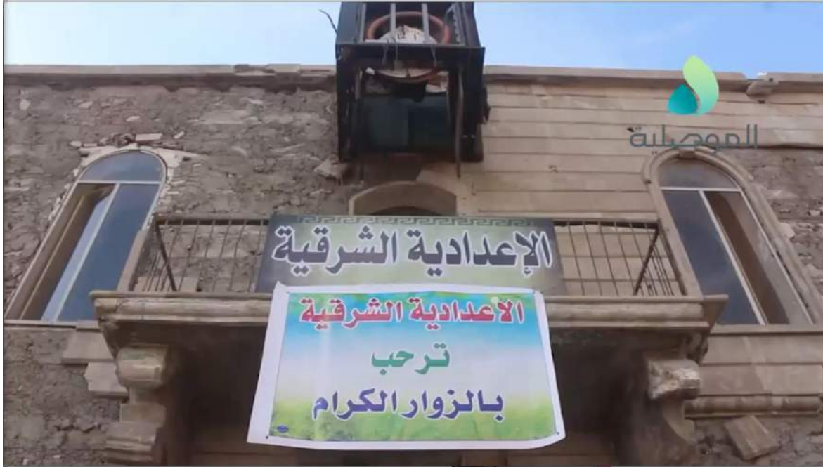
Video still of damage to the exterior of the Eastern Preparatory School (al-Mosuliya; December 15, 2017)
