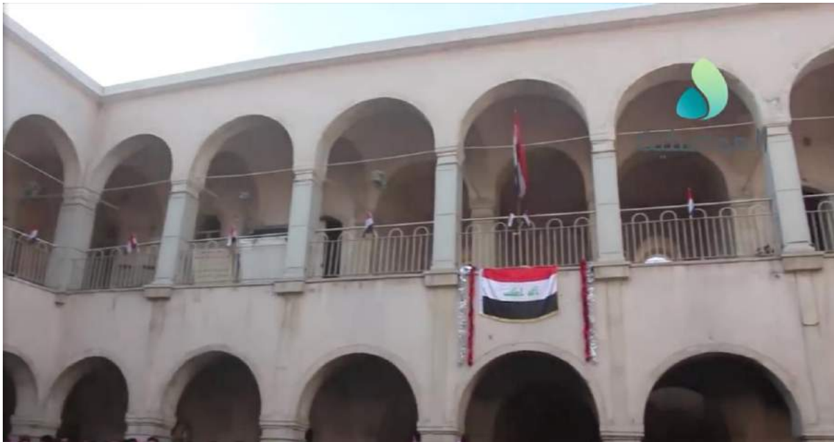
Video still of damage to interior courtyard of the Eastern Preparatory School (al-Mosuliya; December 15, 2017)
