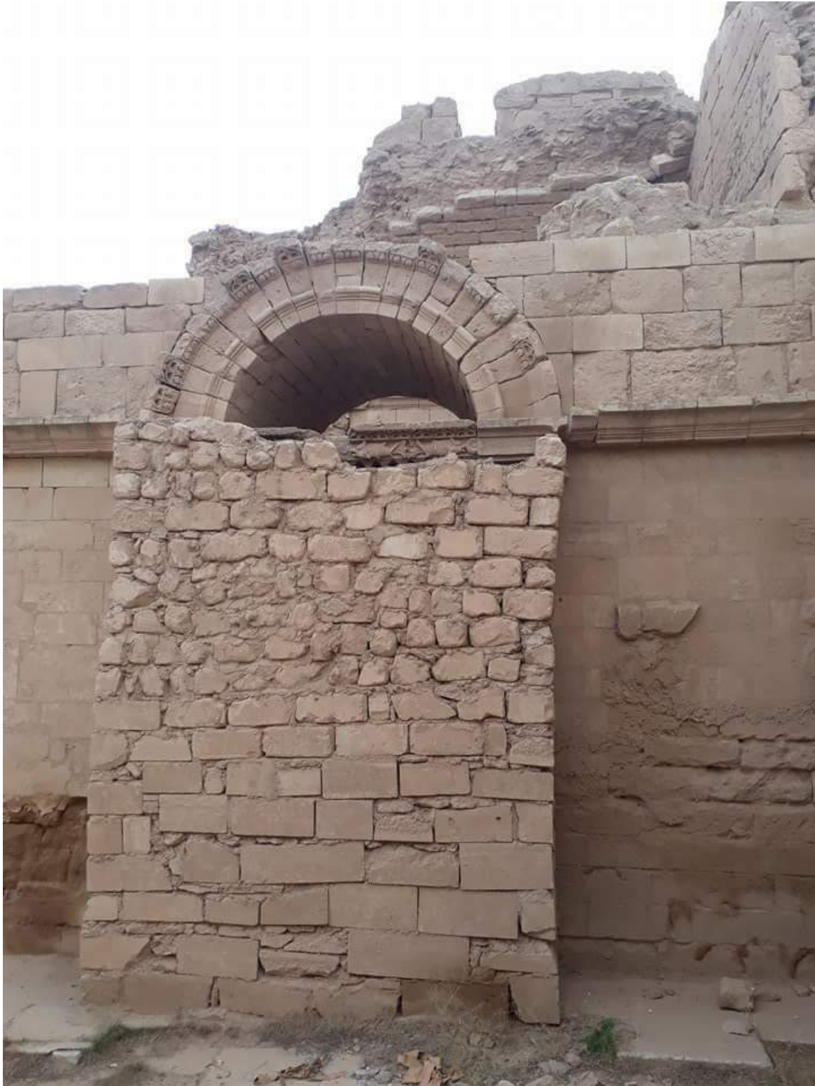
Damage to a buttress at Hatra, due to weathering and neglect (ASOR CHI Source; December 14, 2017)
