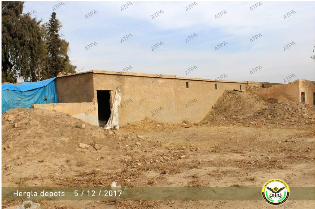
The current condition of the storage facility, seen from the southwest (ATPA; December 11, 2017)
