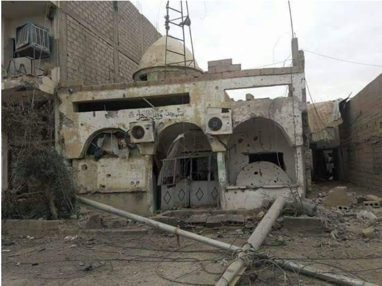
The condition of Fatima al-Zahra Mosque (Euphrates Post; November 29, 2017)
