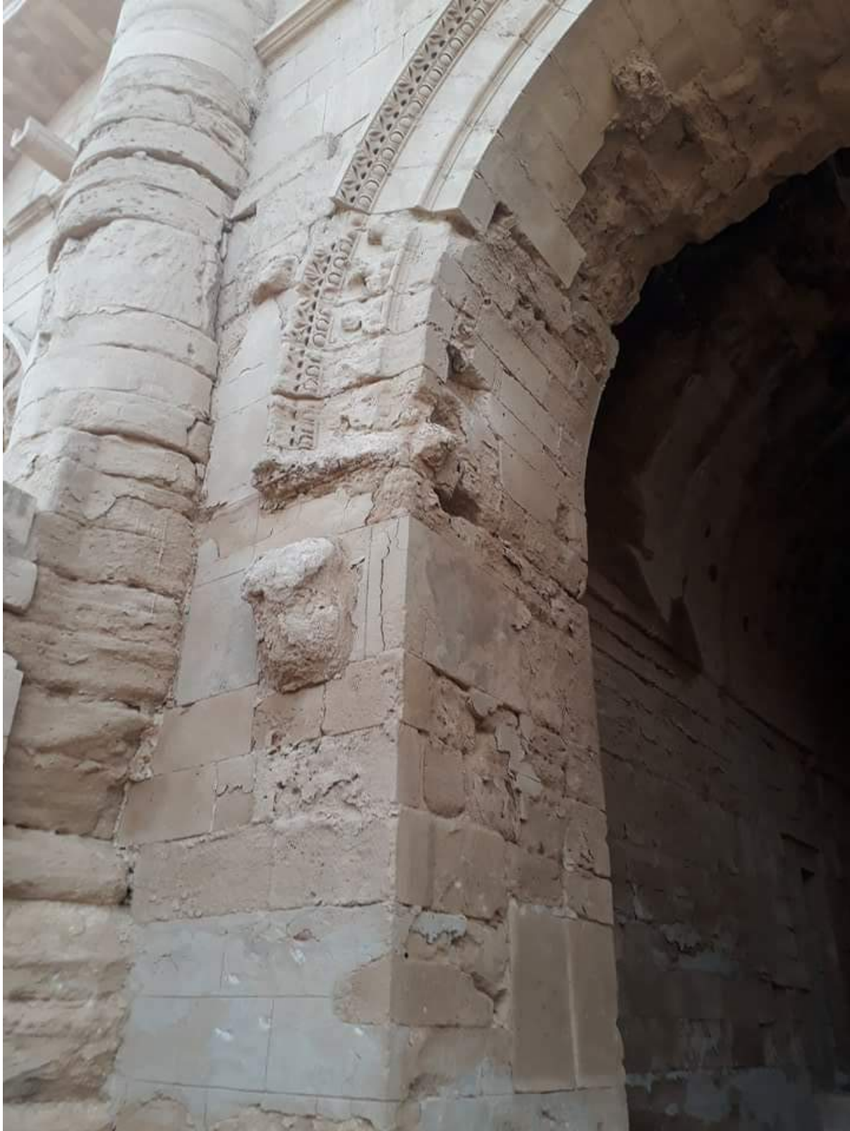
Damage to a gateway from gunfire/shrapnel and damage to a face either intentional or due to weathering (ASOR CHI Source; December 14, 2017)
