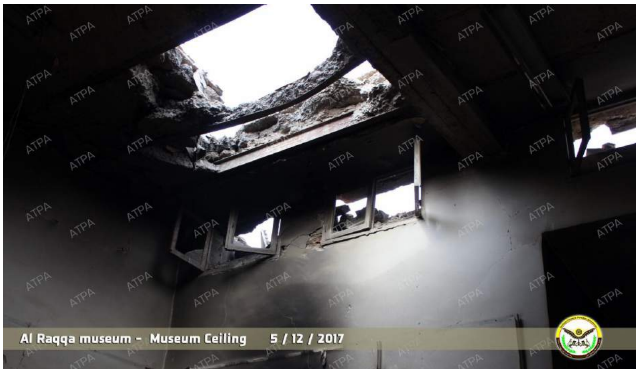
The hole in the roof in the northwestern corner of the central hall on the second floor, seen from the southeast (ATPA; December 11, 2017)
