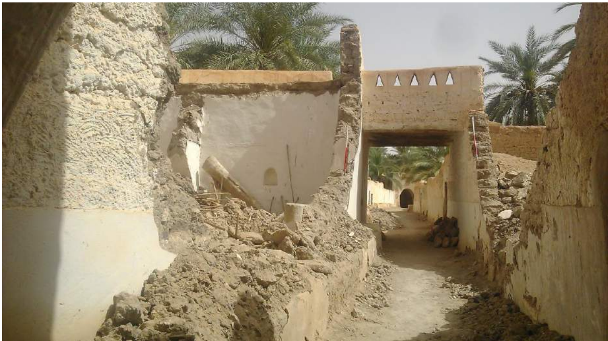
An exterior view of the collapsed school (Hassan Hamoudeh; April 4, 2018)
