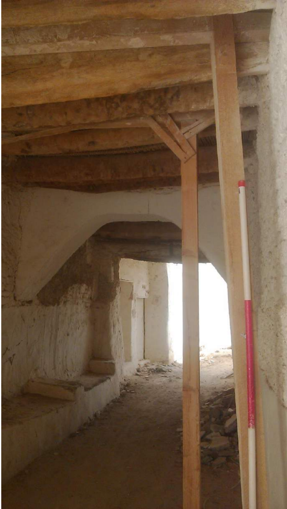
The entrance passage of this house showed signs of collapse and has been stabilized with provisional shoring (Hassan Hamoudeh; April 4, 2018)
