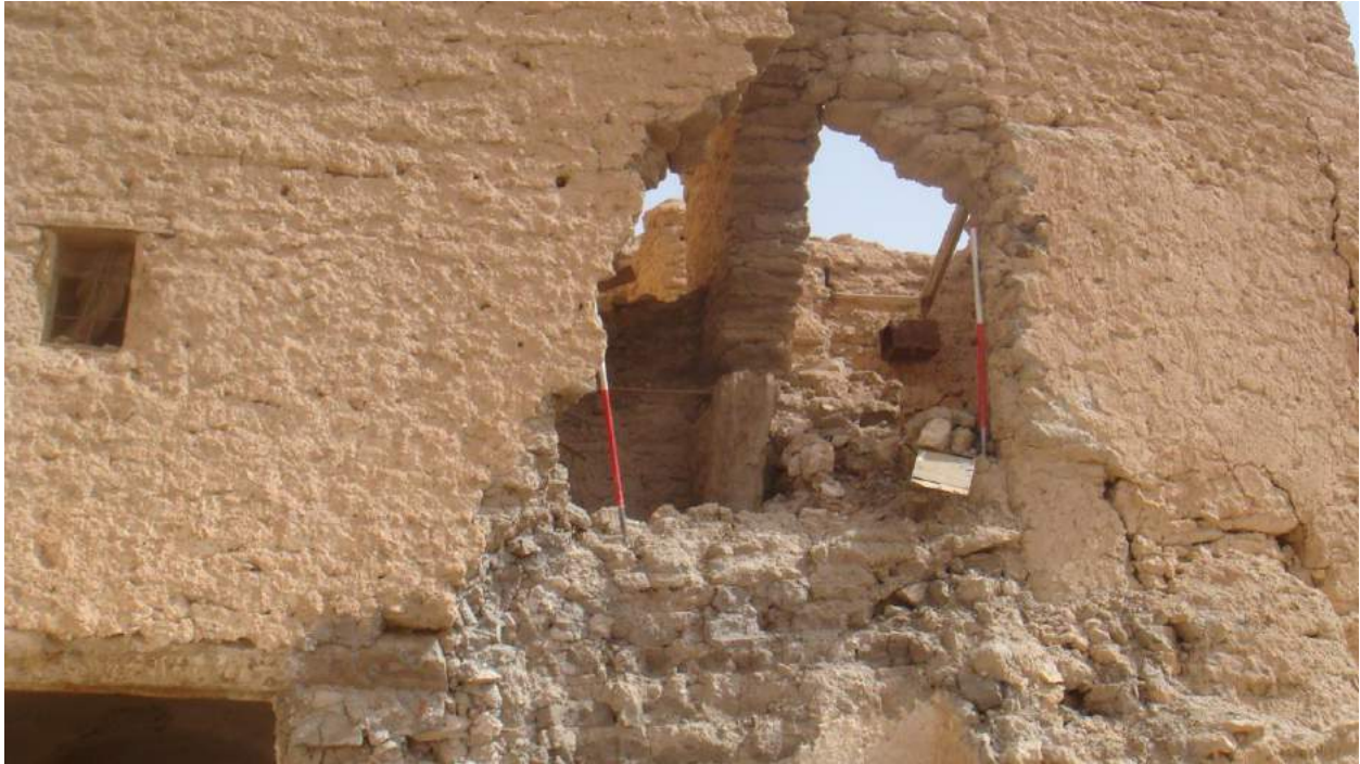
A close-up view of the collapse of a section of a wall at Location 3 (Hassan Hamoudeh; April 4, 2018)
