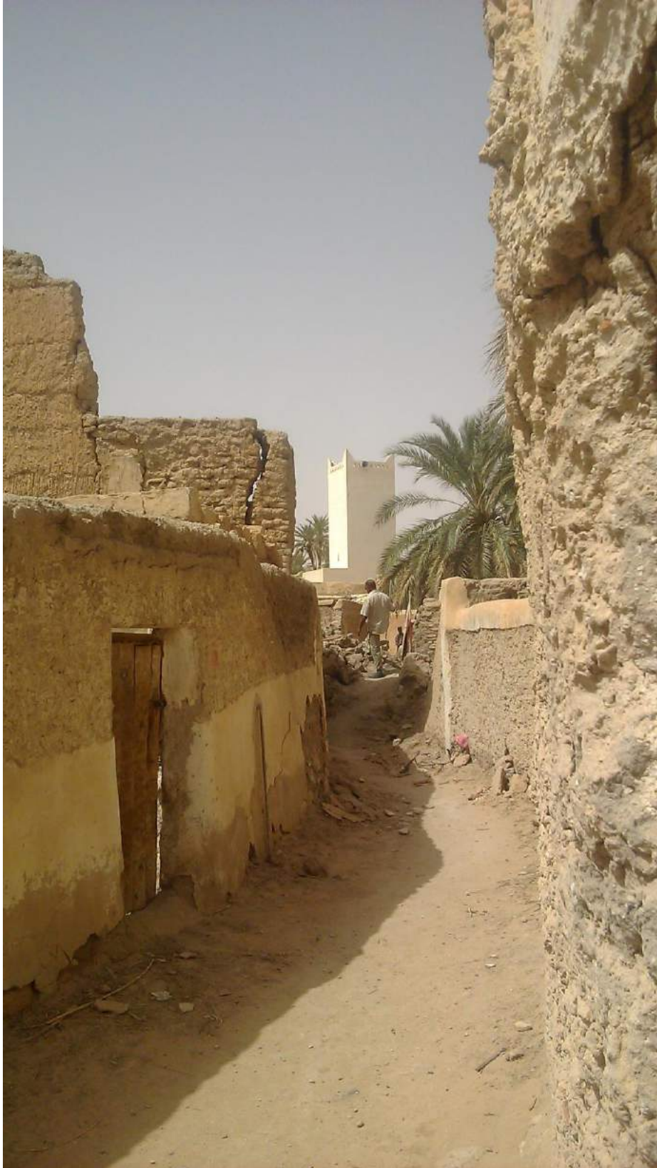
Some of the walls at Location 5 remain standing but have separated entirely from other nearby walls, suggesting that collapse is imminent (Hassan Hamoudeh; April 4, 2018)
