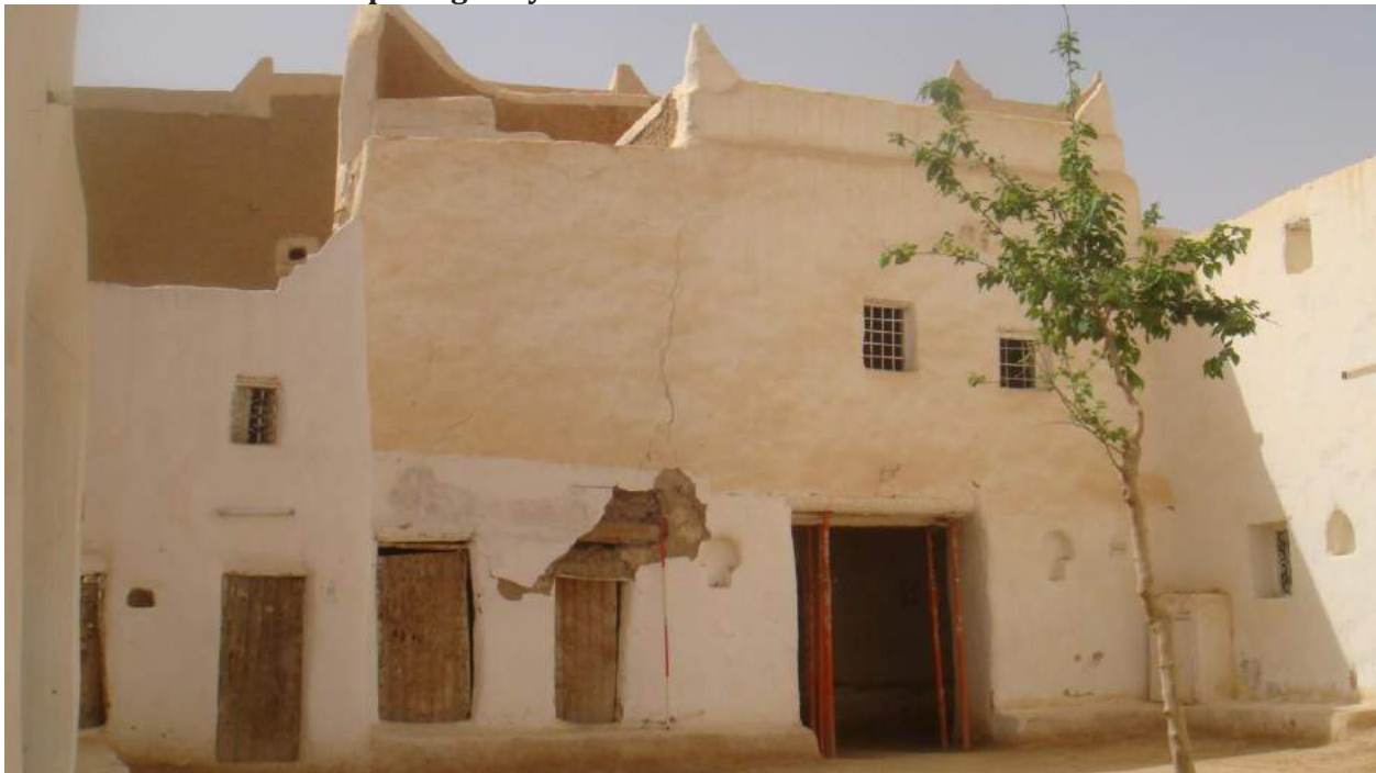
Damage to an exterior wall and entranceway at Location 4 (Hassan Hamoudeh; April 4, 2018)
