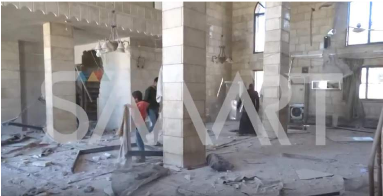
Damage to the interior of al-Rahman Mosque (SMART News Agency; April 5, 2018)
