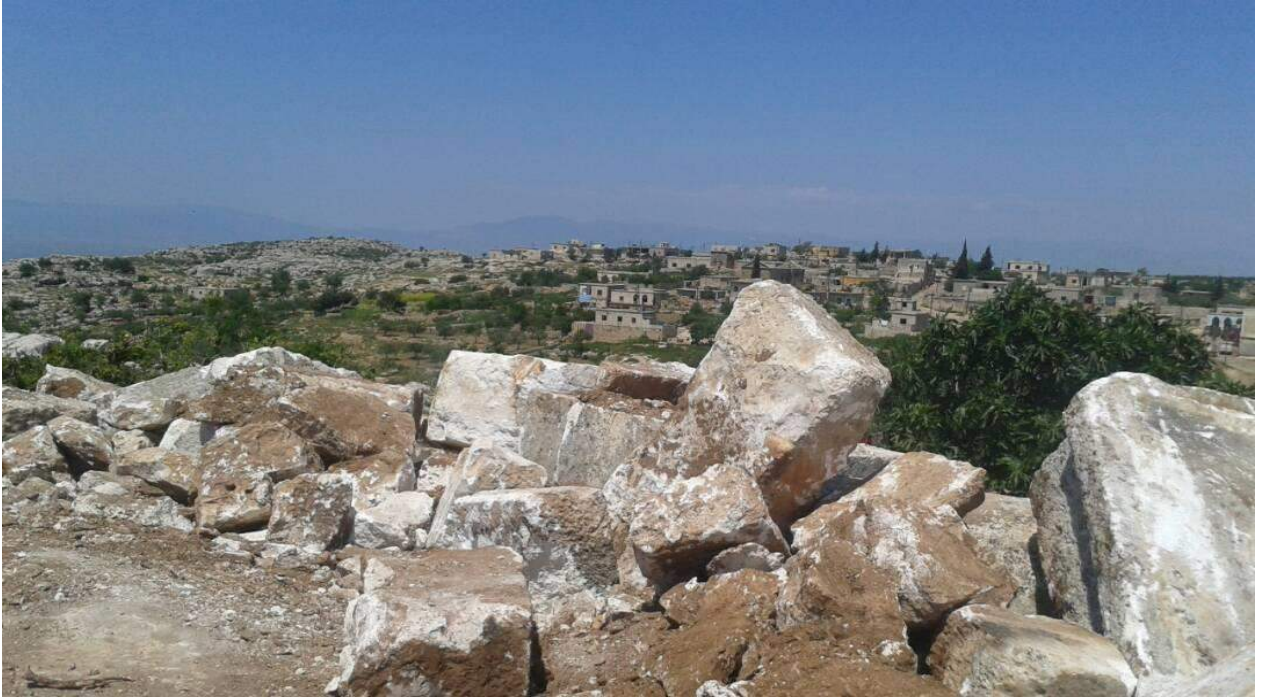
Damaged stone masonry
