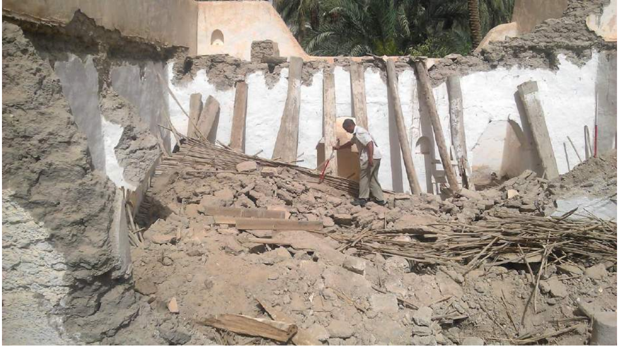
A DoA Ghadames employee examines the damage to the collapsed roof of the school. Many of the timbers remain intact (Hassan Hamoudeh; April 4, 2018)
