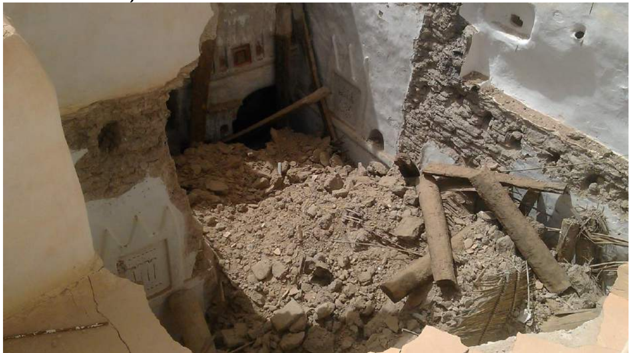
A view of Location 1, where portions of two adjacent houses separated by a partition wall have collapsed. Date palm trunks and woven mats that once supported the floors and roof can be seen in the debris pile (Hassan Hamoudeh; April 4, 2018)
