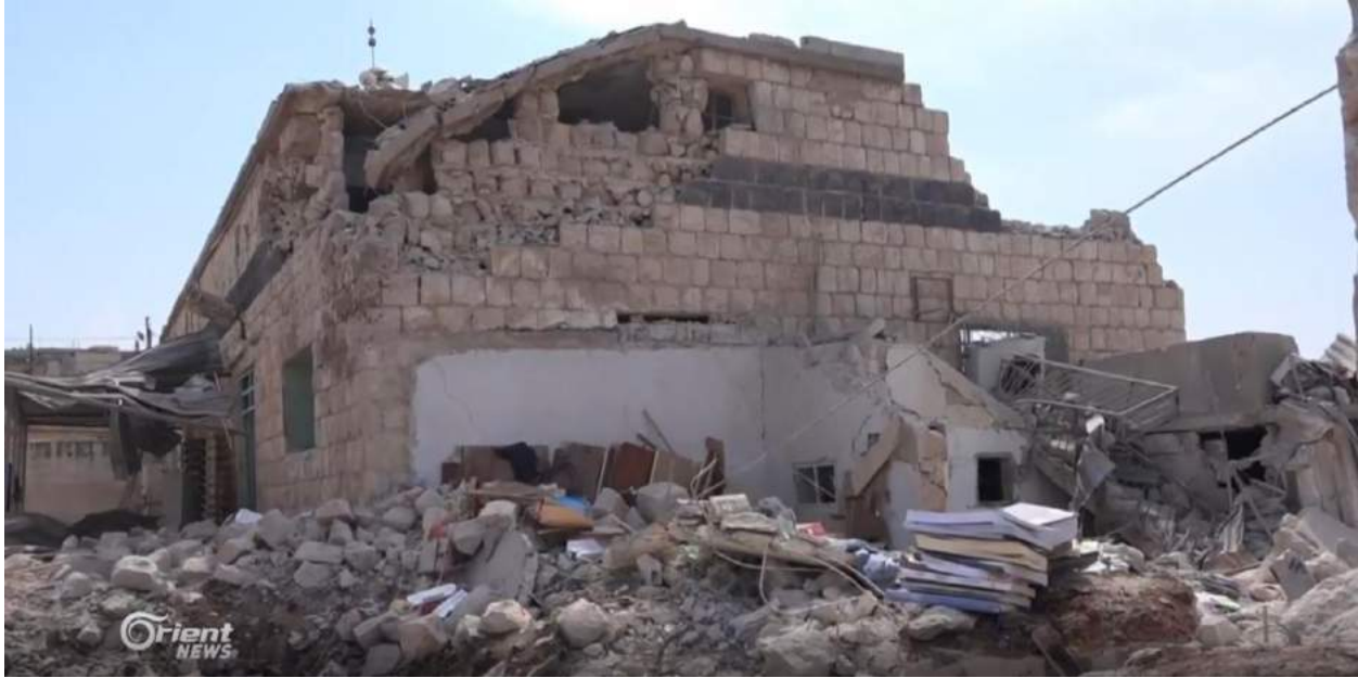
Damage to al-Kabir Mosque (Orient News; April 30, 2018)
