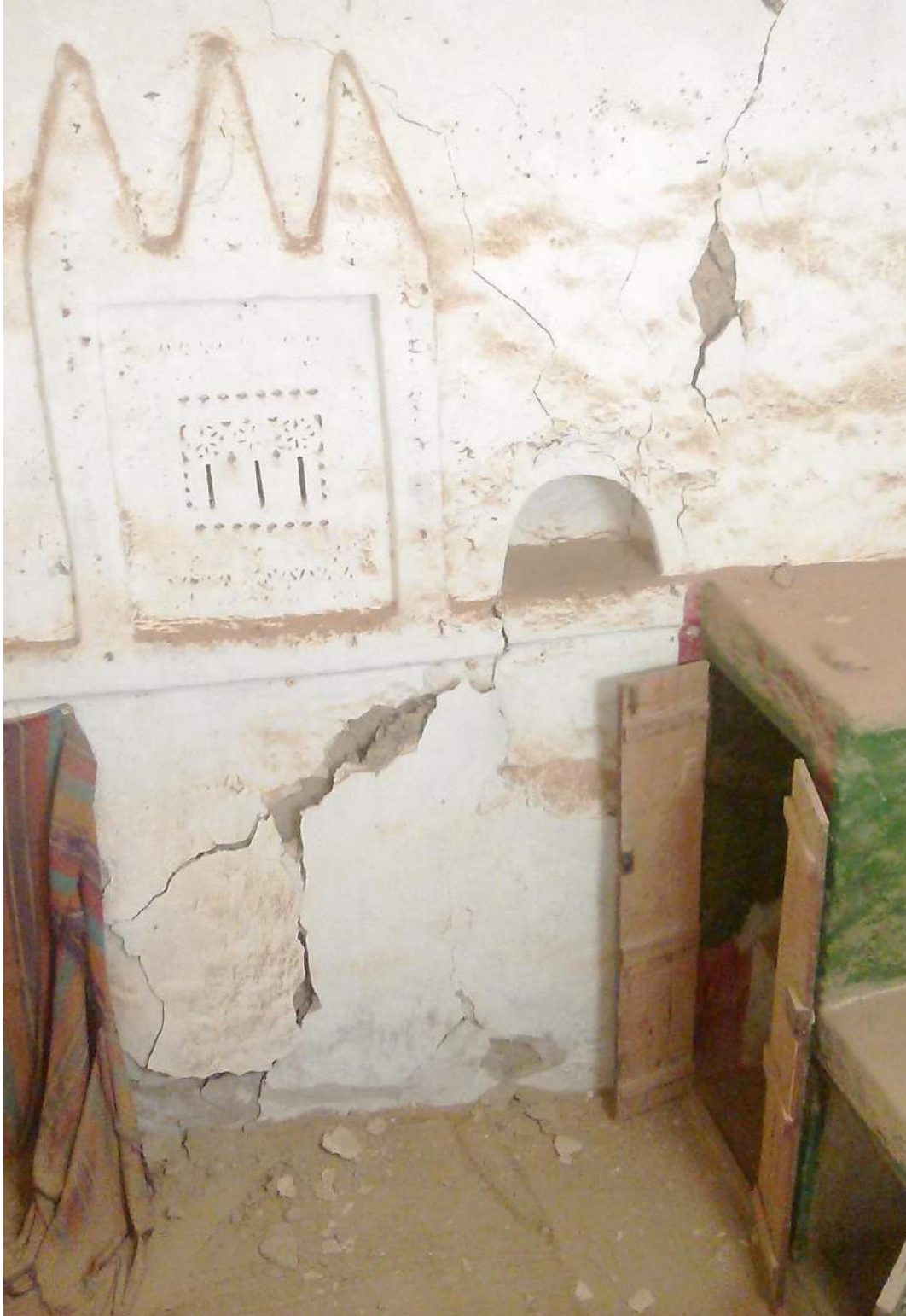
The interior of one of the two houses at Location 1. Cracks have proliferated in the lime plaster of this wall, suggesting that the earthen mass behind it has started to shift and may soon collapse (Hassan Hamoudeh; April 4, 2018)
