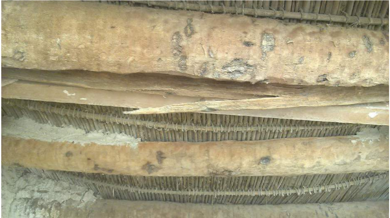
A view of the palm wood supports in the passageway near Location 4, which are beginning to buckle and crack (Hassan Hamoudeh; April 4, 2018)
