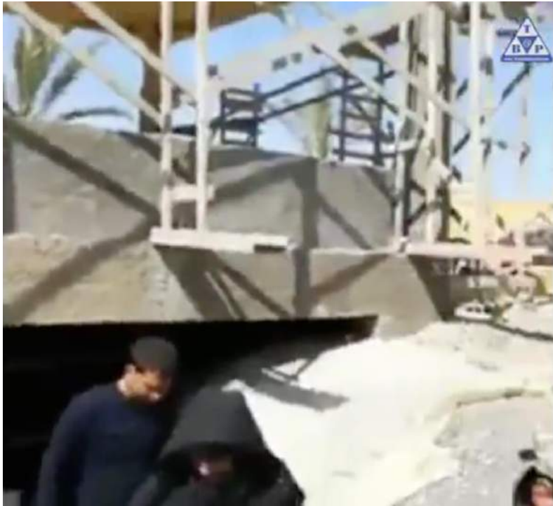
Video still of the shrine during its construction, seen from the southeast (Baghdad Post; April 24, 2018)
