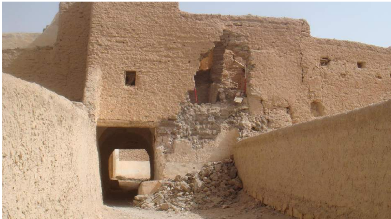
Sections of collapse, like those at Location 3, may be stabilized using infill of adobe brick. If such actions are taken swiftly, it is possible to save the structure as a whole (Hassan Hamoudeh; April 4, 2018)
