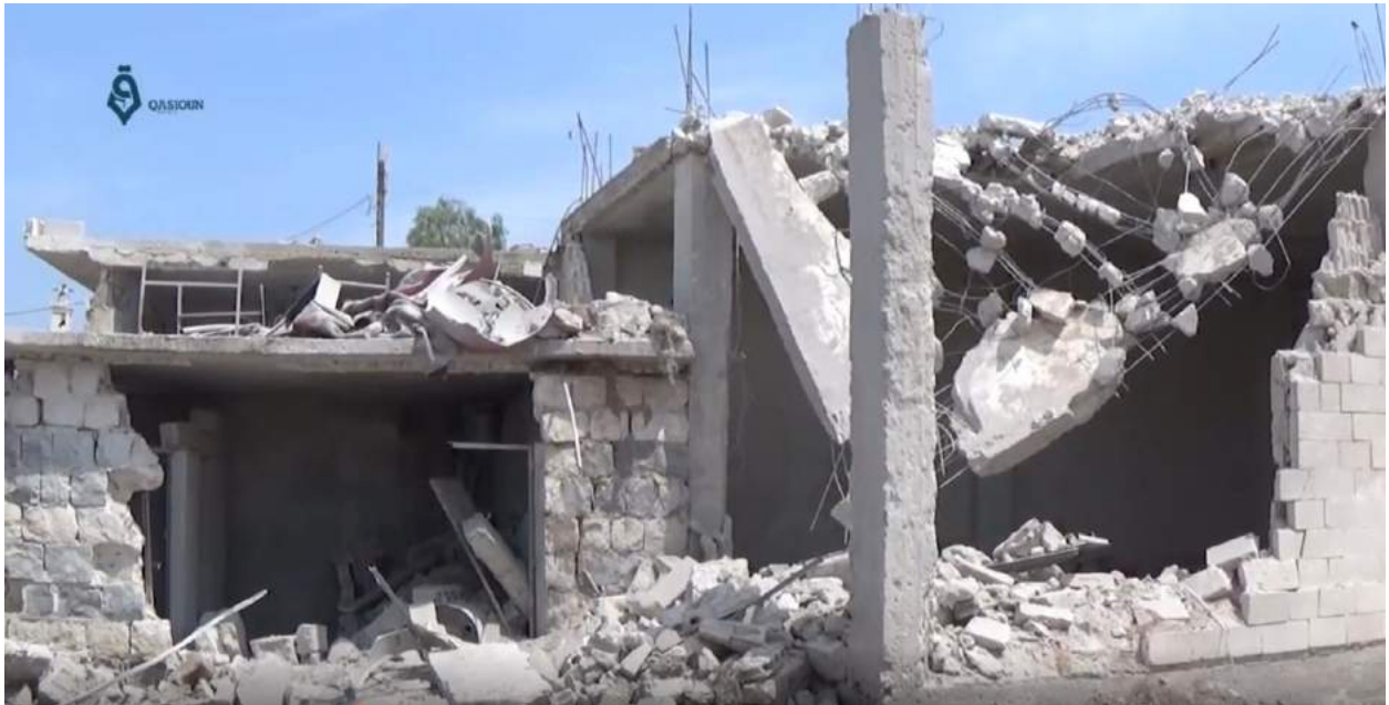
Damage to the roof of al-Kabir Mosque (Qasioun News Agency; April 30, 2018)
