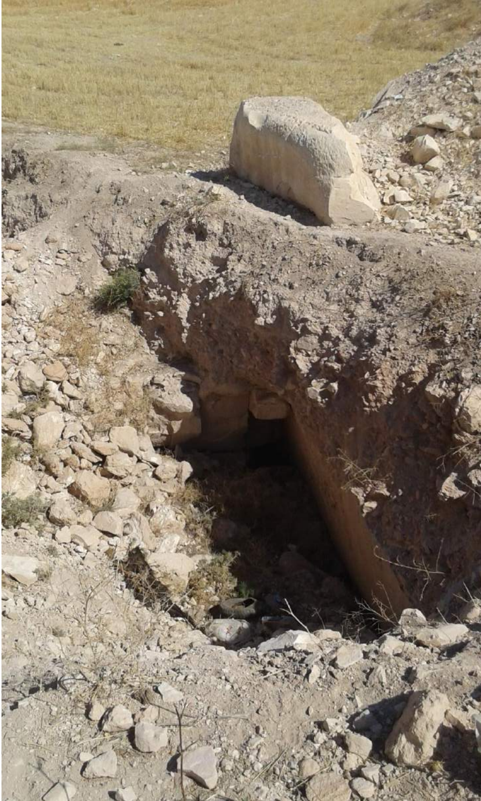
An illegal excavation shows some old foundation
