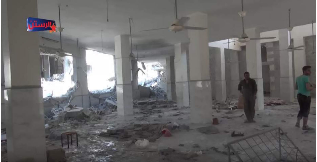
Damage to the interior of al-Omari Mosque (Suhaib al-Ali - Homs; April 30, 2018)
