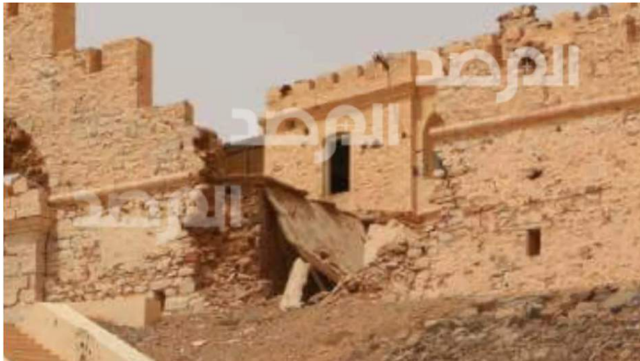
Collapse of a section of southern wall of Sabha Castle to right side of entrance (Al Marsad; April 1, 2018)
