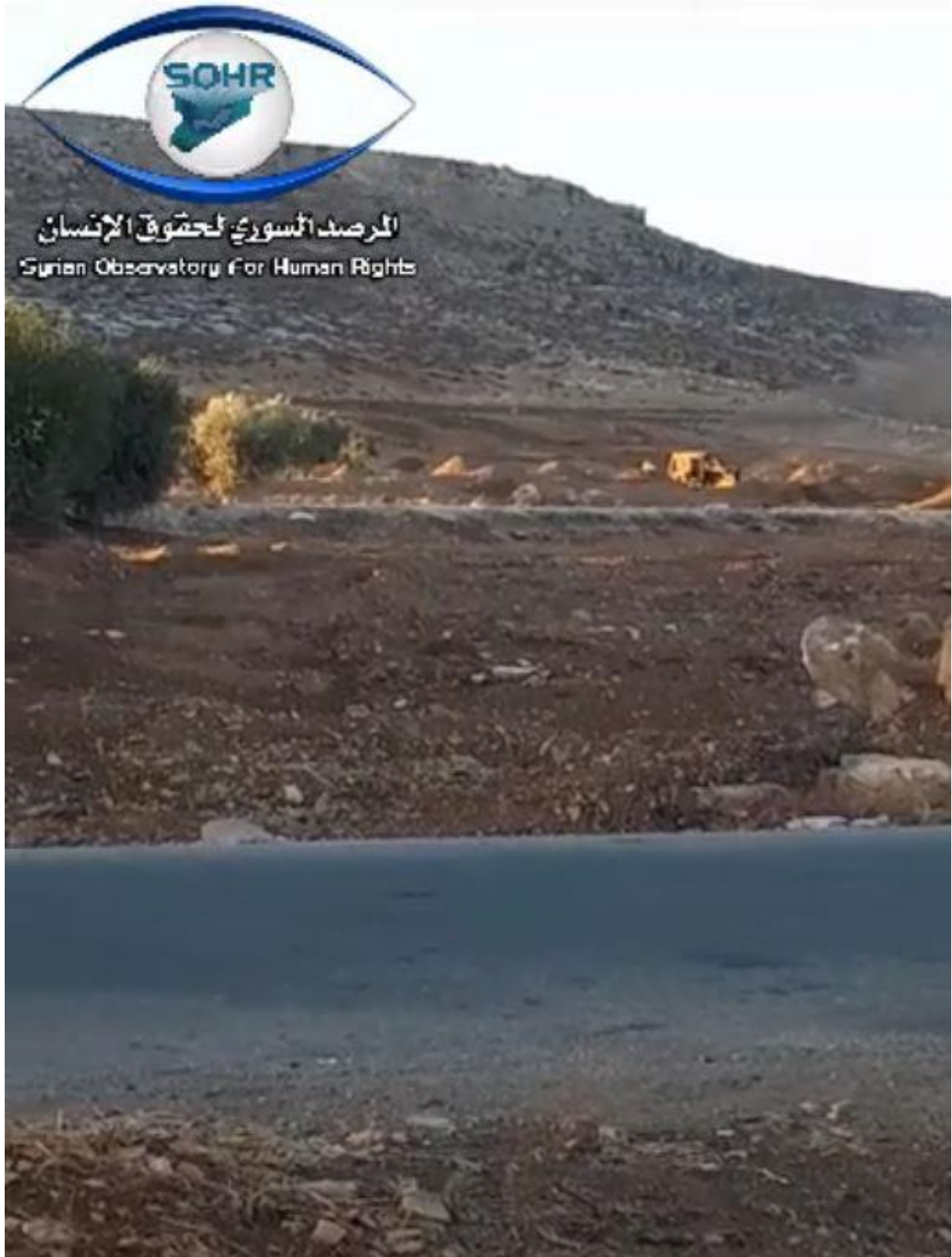
Video still of an earth mover working on the archaeological site of Cyrrhus (SOHR; October 2, 2018)
