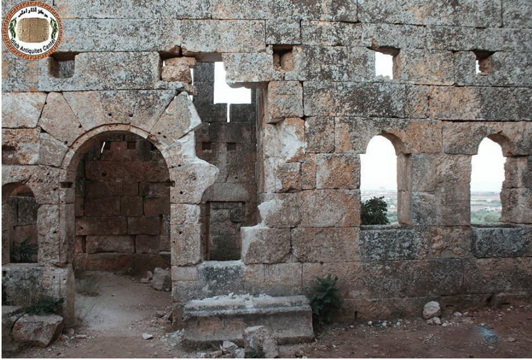
The facade of Deir Sobat showing damage due to possible gunfire and/or looting and vandalism of stones (Idlib Antiquities Center; July 14, 2018)
