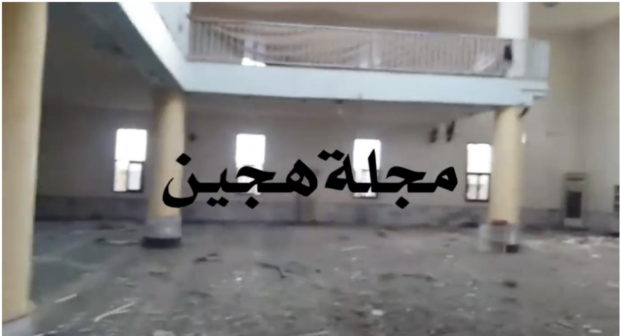
Video still of the interior of the mosque, seen from the west (Majlat Hajin; December 7, 2018)
