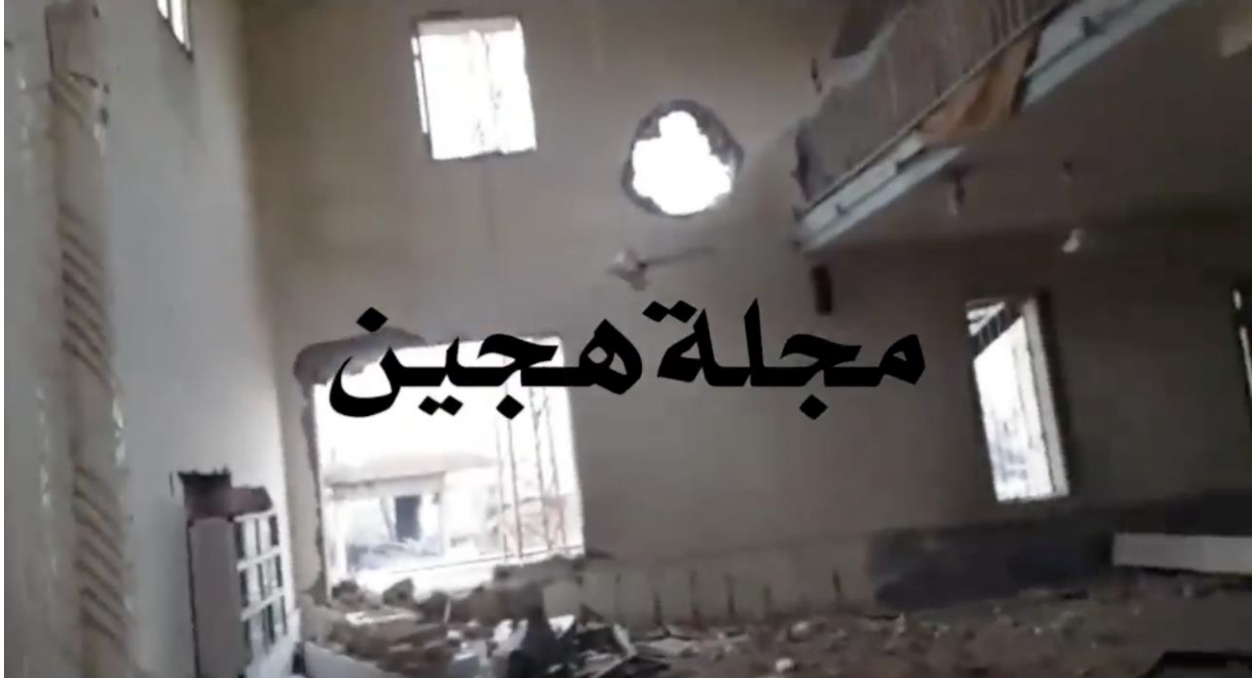
Video still of the damage to the mosque, seen from the east (Majlat Hajin; December 7, 2018)
