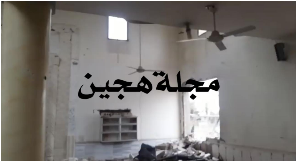
Video still of damage to the southwest corner of the mosque (Majlat Hajin; December 7, 2018)
