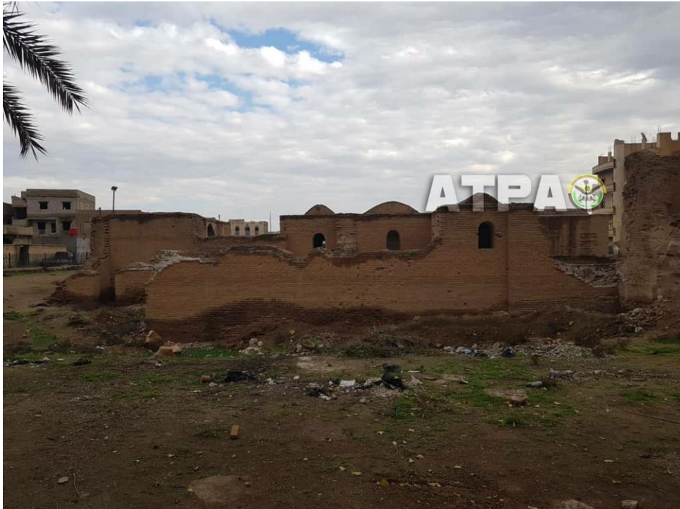
Moisture in the walls of Qasr al-Banat (ATPA; December 14, 2018)
