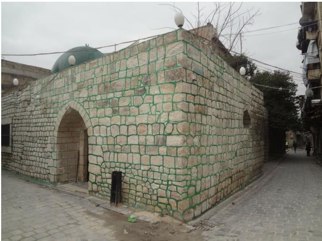
The reconstructed corner of al-Akhal Mosque with green mortar (Middle East Eye; December 16, 2018)
