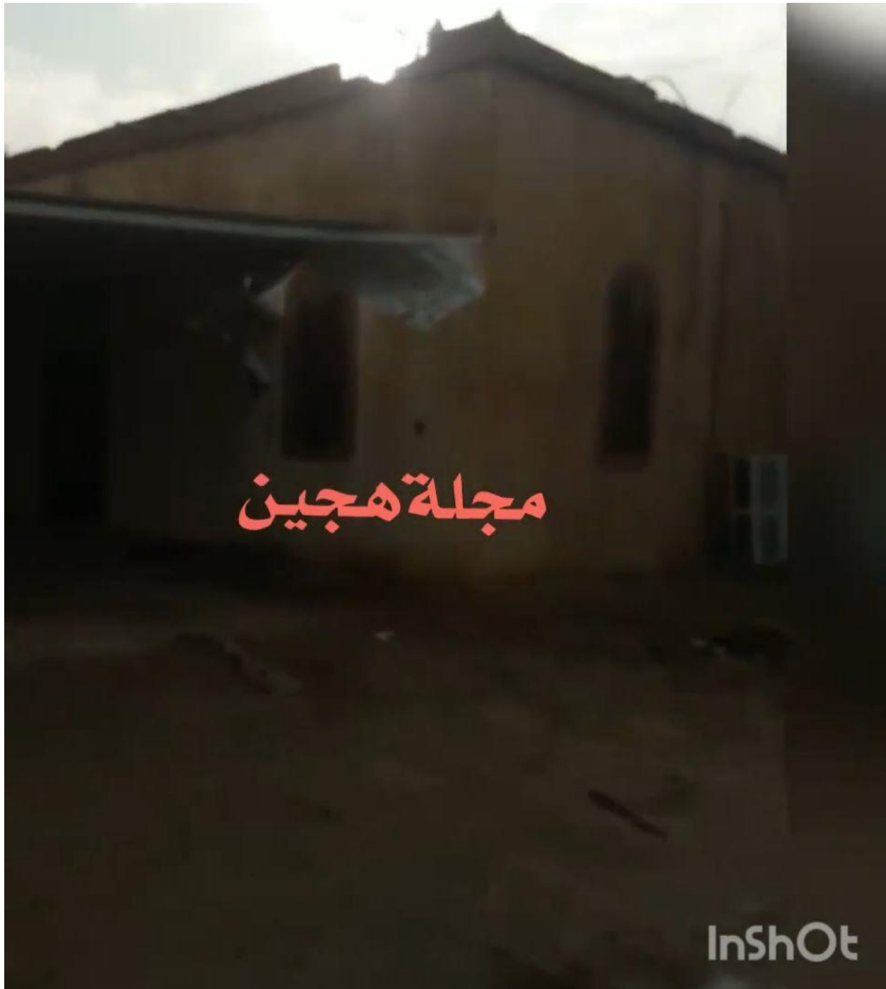
Video still of the northwestern corner of the mosque; note the damage to the upper corner and the aluminum roof in front of the mosque (Majlat Hajin; December 20, 2018)
