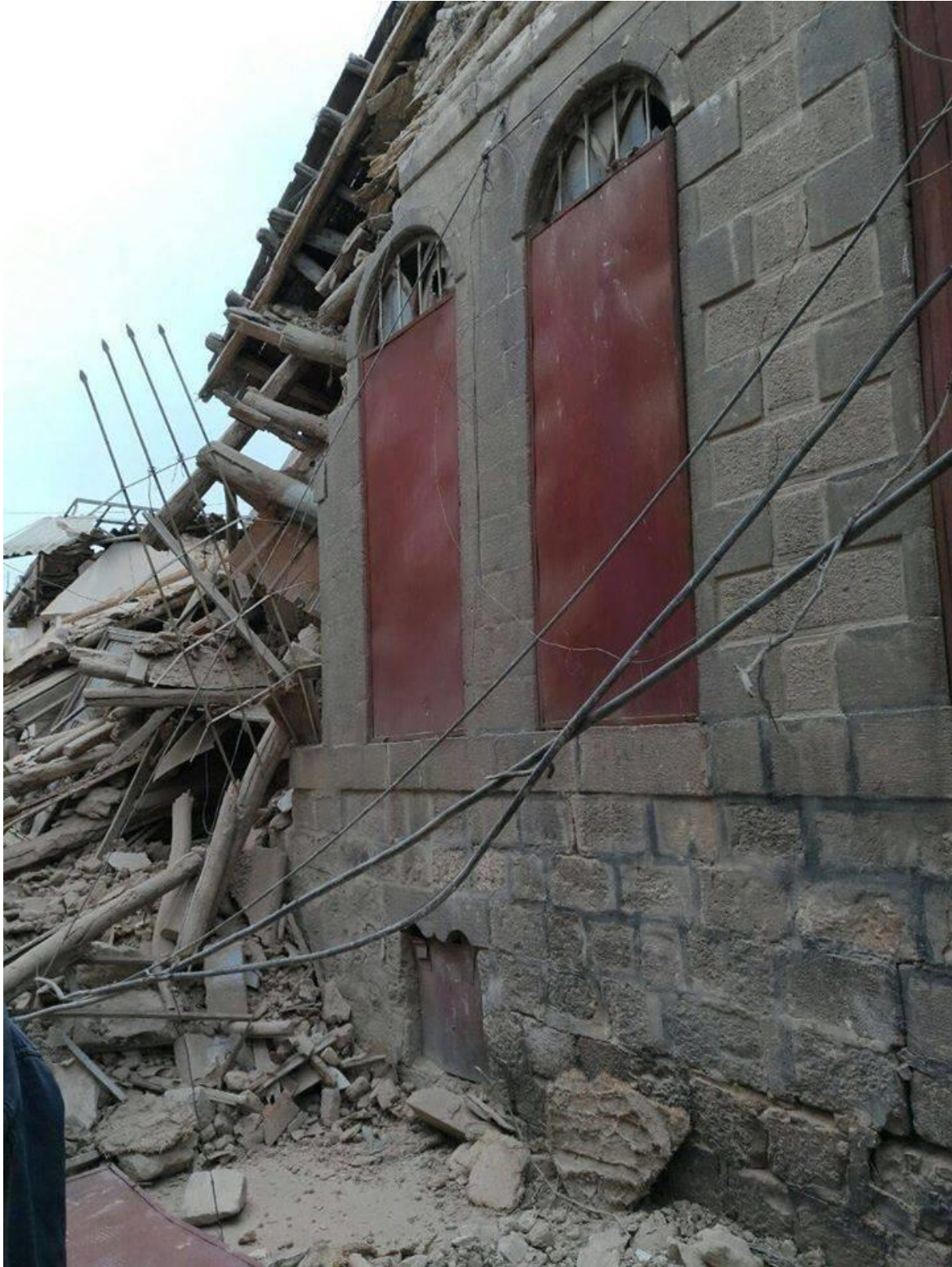
The side of the collapsed house (Damascus Now; December 15, 2018)
