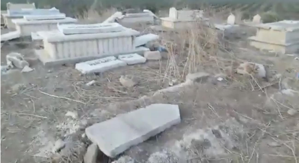
Video still of widespread damage to the cemetery (Private Twitter Account; December 11, 2018)
