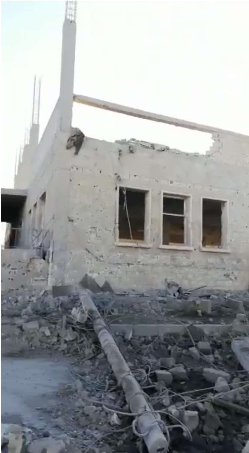
Video still of damage to the northwestern corner of the mosque, seen from the west (Majlat Hajin; December 12, 2018)
