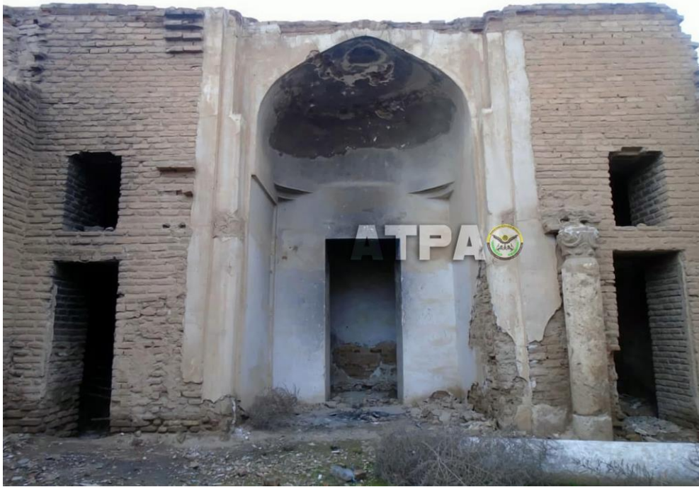
The current condition of an iwan in the palace; note the loss of plaster near the base of the walls (ATPA; December 14, 2018)
