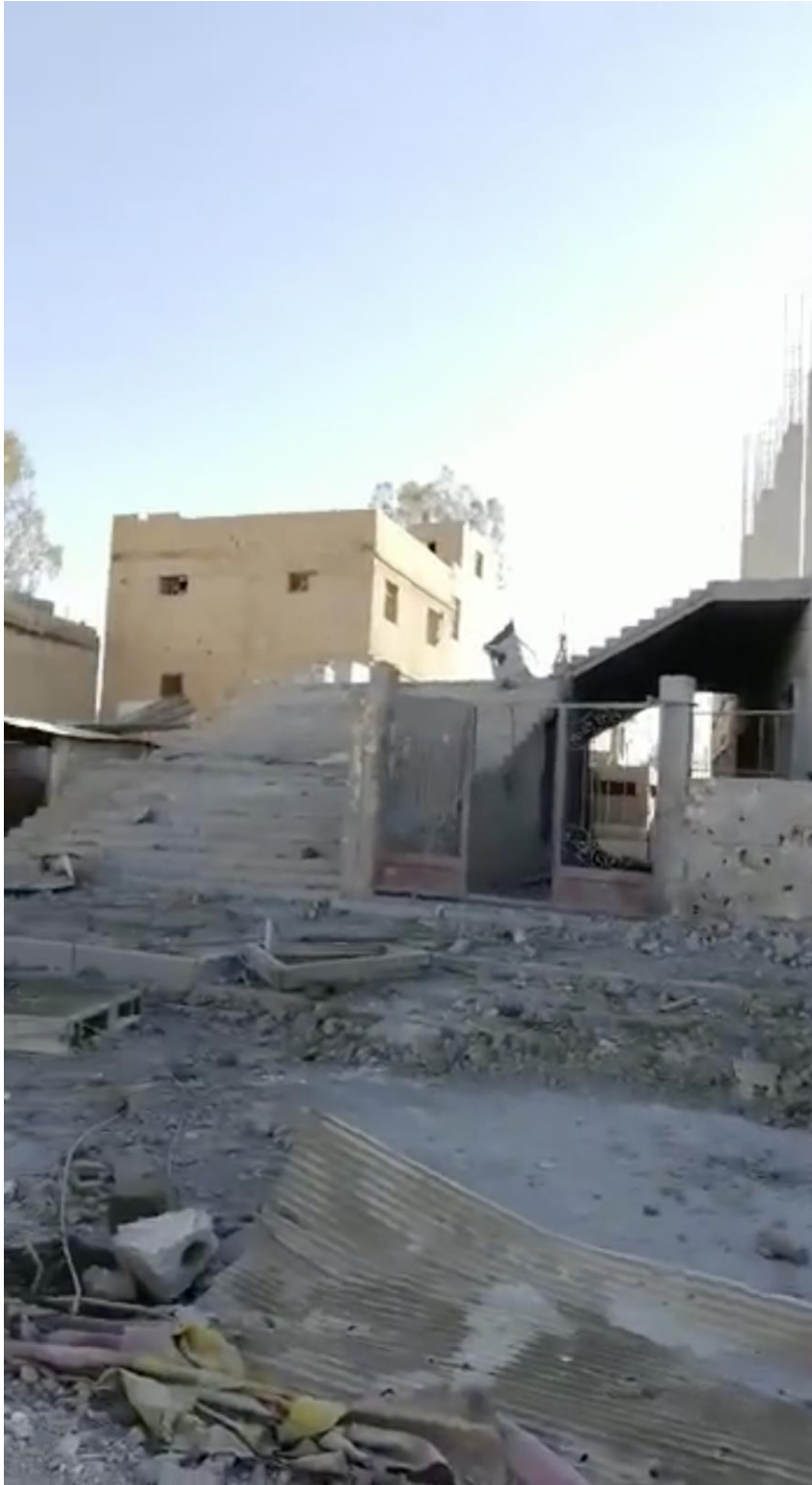
Video still of a stairway to the northern end of the unfinished second story of the mosque, seen from the west (Majlat Hajin; December 12, 2018)
