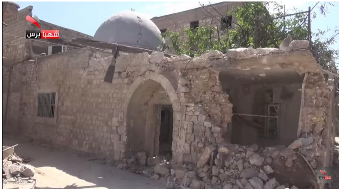
Video still of damage to the mosque (Shaba Press; May 1, 2015)
