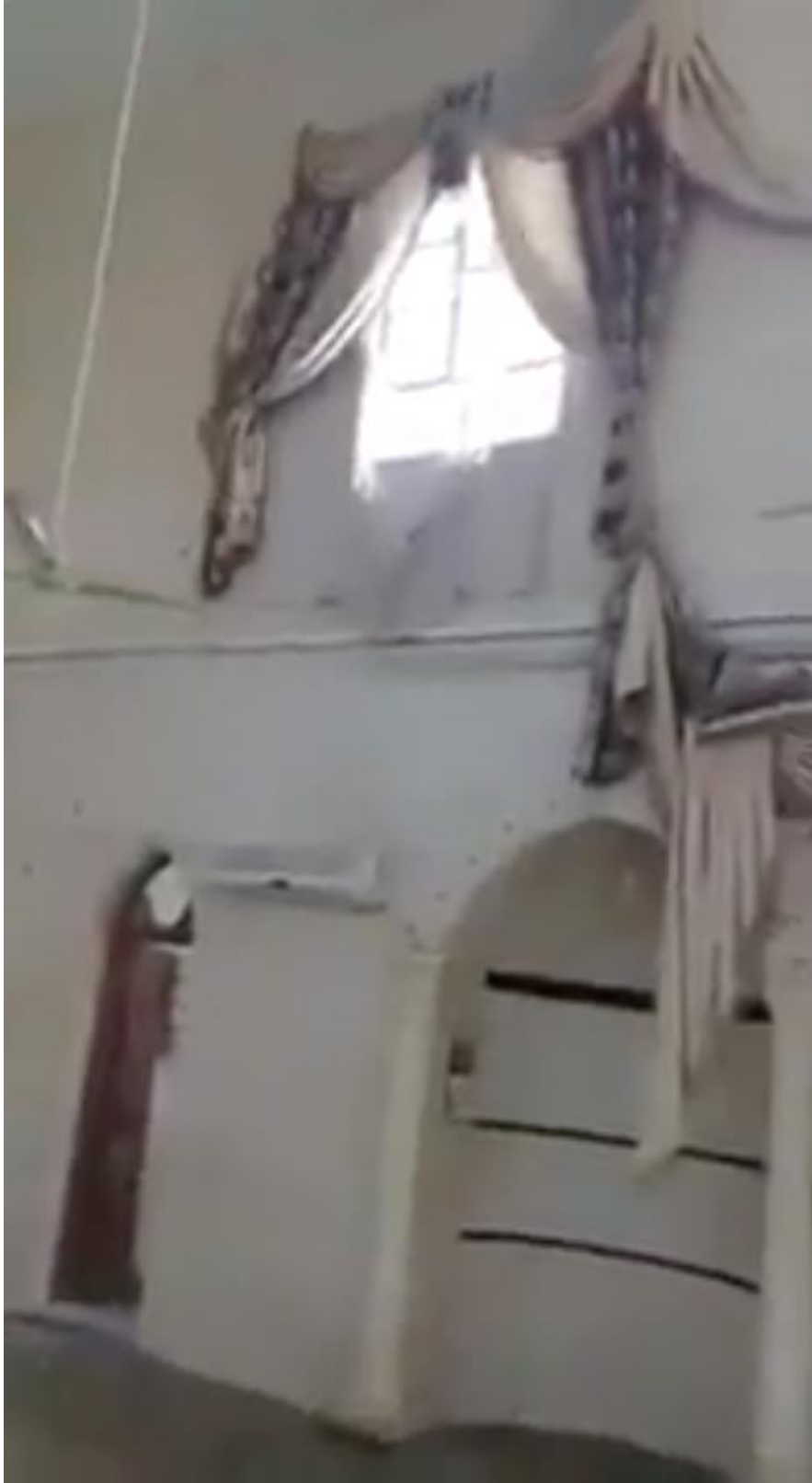
Video still showing damage to the Khalid bin al-Walid Mosque (SNHR; August 23, 2018)
