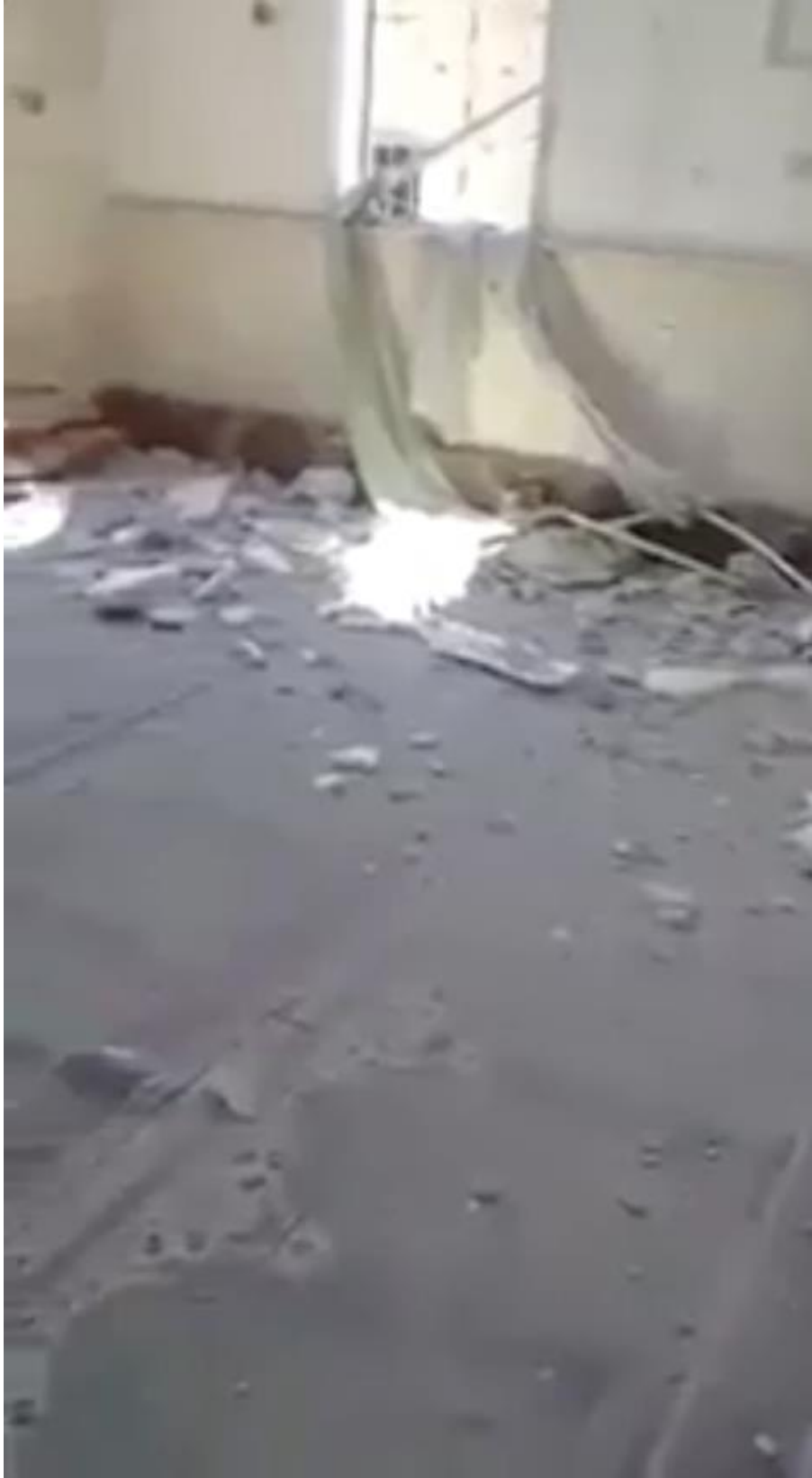
Video still showing damage to the Khalid bin al-Walid Mosque (SNHR; August 23, 2018)
