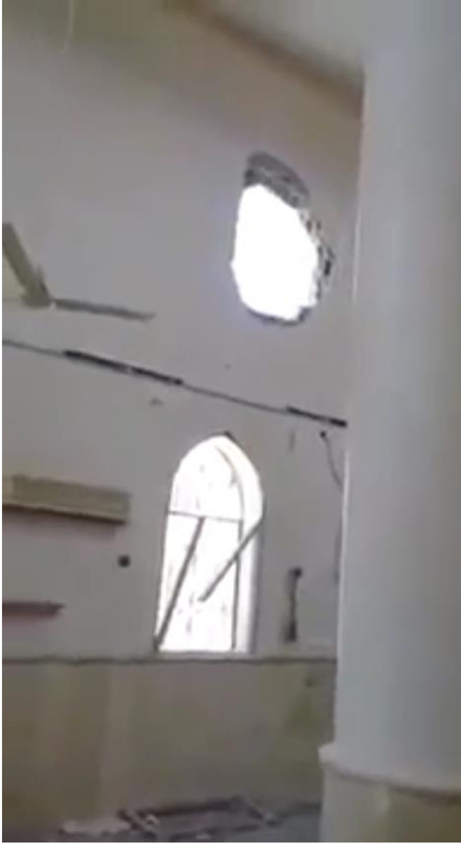
Video still showing damage to the Khalid bin al-Walid Mosque (SNHR; August 23, 2018)
