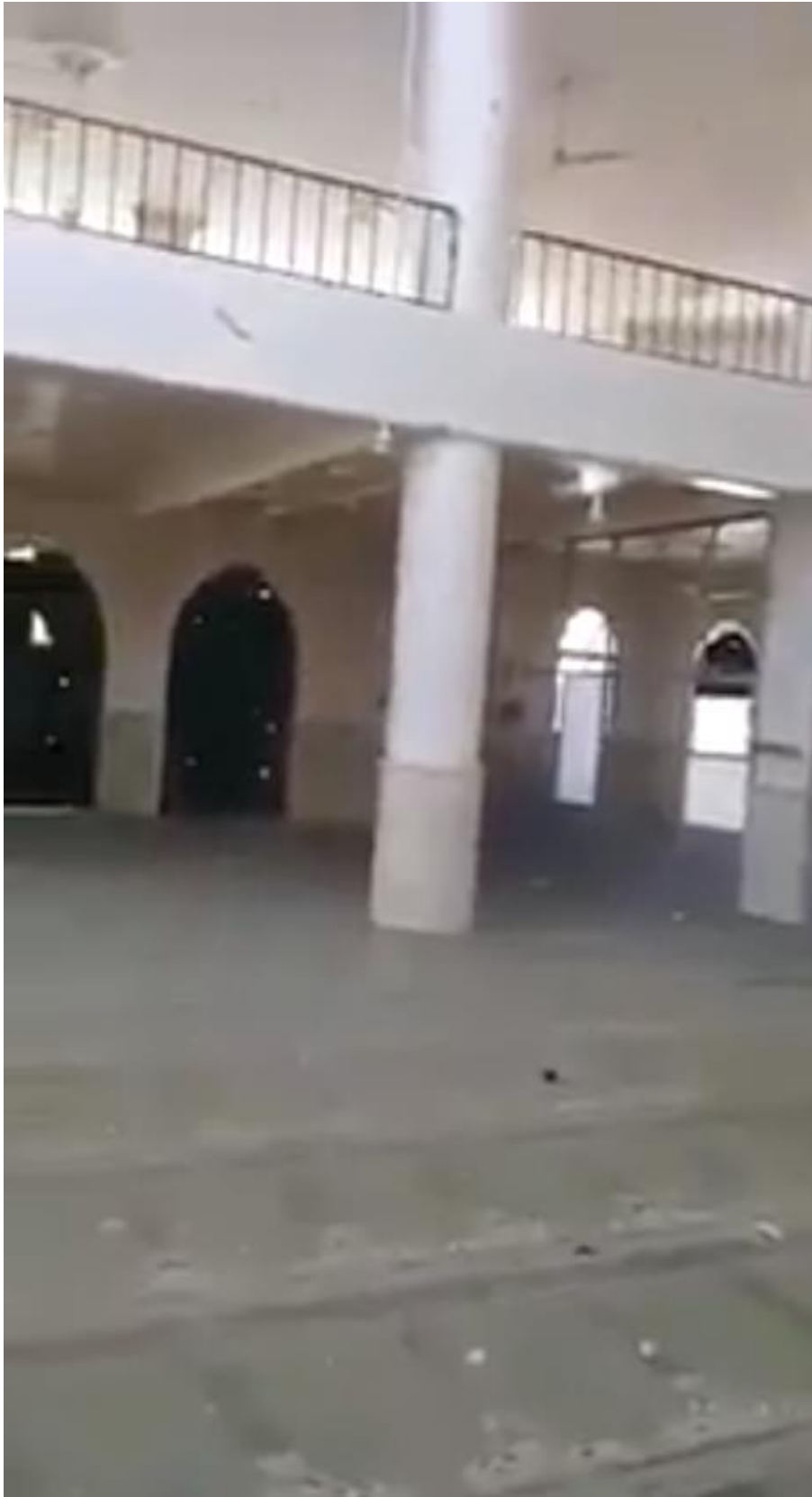
Video still showing damage to the Khalid bin al-Walid Mosque (SNHR; August 23, 2018)
