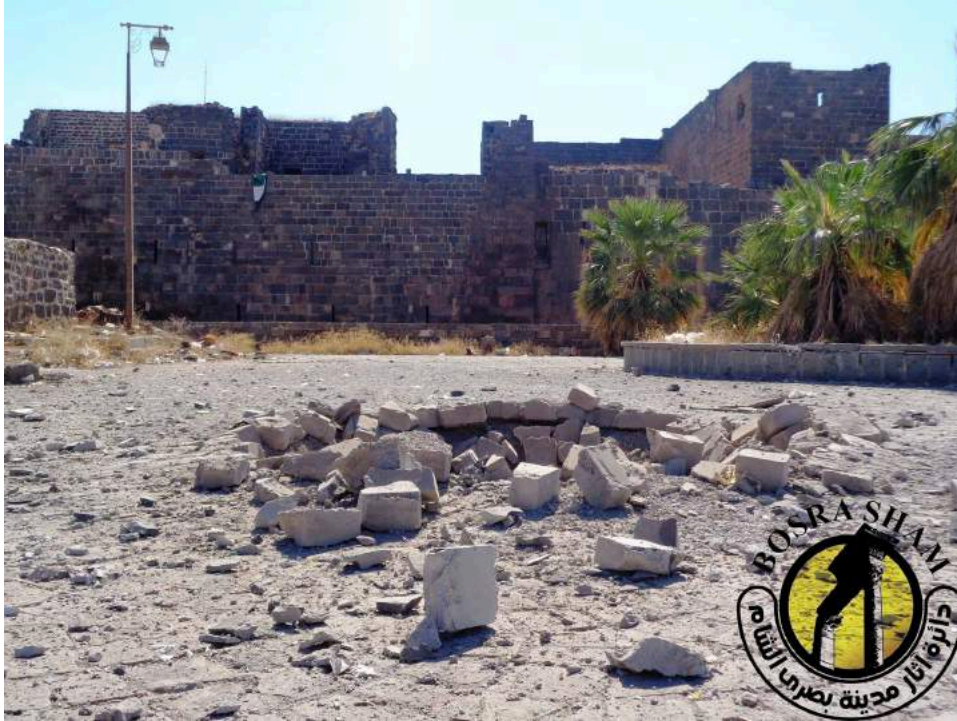
Busra al-Sham Citadel Courtyard showing bomb damage (Facebook; September 16, 2015)
