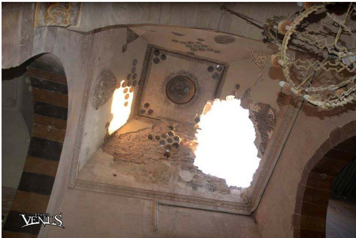
The Armenian Catholic Cathedral Our Lady of Pity, Aleppo, damage to the dome caused by mortar fire. (Venus Studio)
