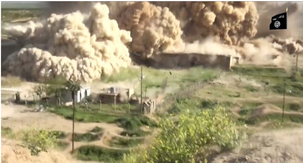
Northwest Palace, Nimrud, Iraq, detonation of the palace (YouTube; screenshot of video posted by ISIL-associated account, showing the demolition of the Northwest Palace)
