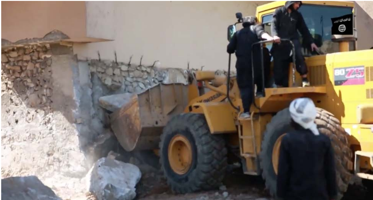
Northwest Palace, Nimrud, Iraq, ISIL militants removing the rubble of the wall relief panels with a bulldozer (YouTube; screenshot of video posted by ISIL-associated account, showing the demolition of the Northwest Palace)
