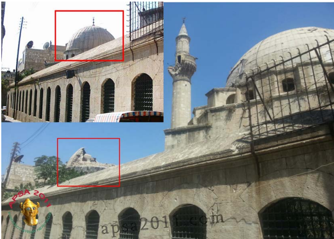
Combat damage sustained to the Madrasa al-'Utmaniya in Aleppo (APSA).
