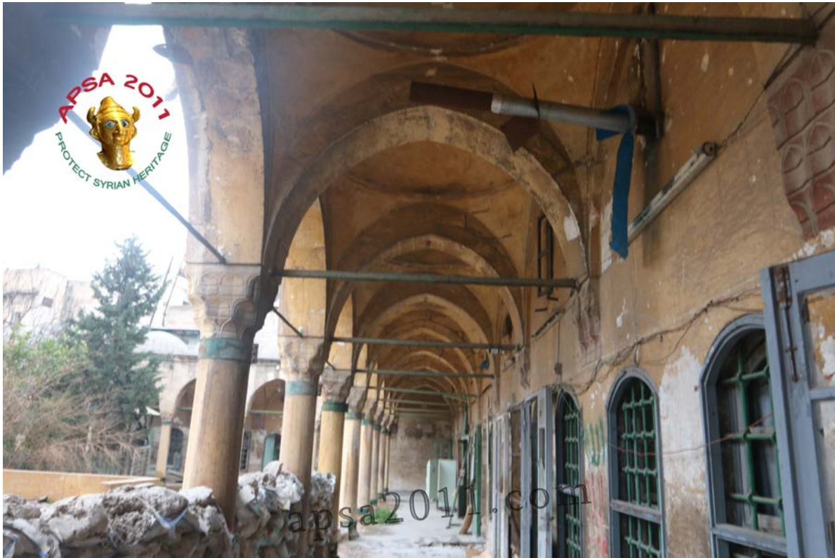
Combat damage sustained to the Madrasa al-'Utmaniya in Aleppo (APSA).
