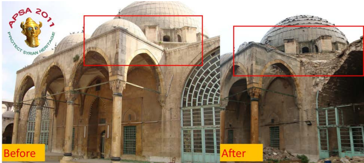
Before- and after-photos of combat damage sustained to the Madrasa al-'Utmaniya in Aleppo (APSA).
