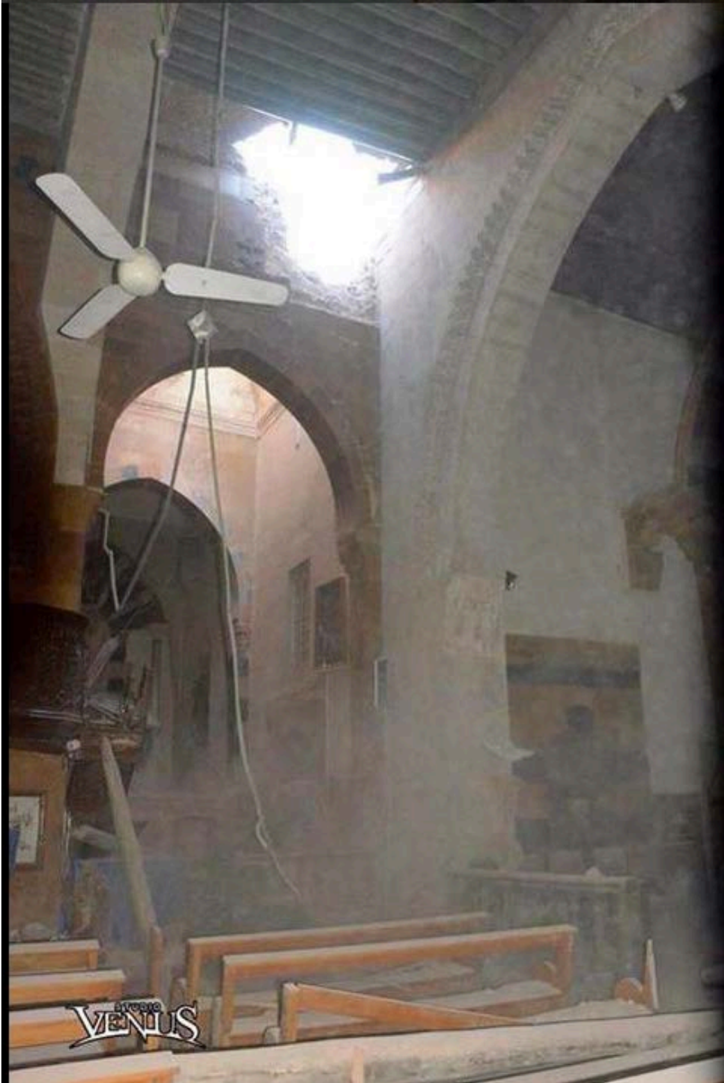
Damage to the interior of the Armenian Catholic Cathedral Our Lady of Pity in Aleppo caused by mortar fire (Venus Studio).
