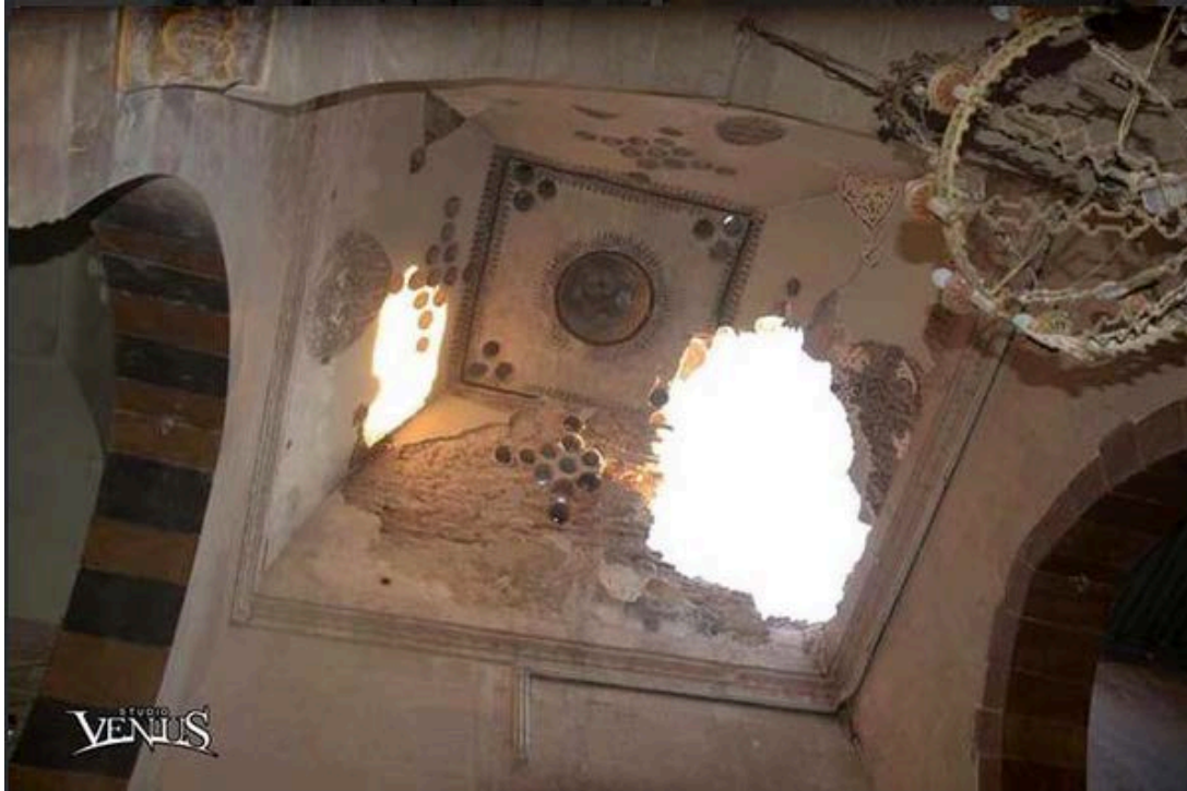
Damage to the dome of the Armenian Catholic Cathedral Our Lady of Pity in Aleppo caused by mortar fire (Venus Studio).
