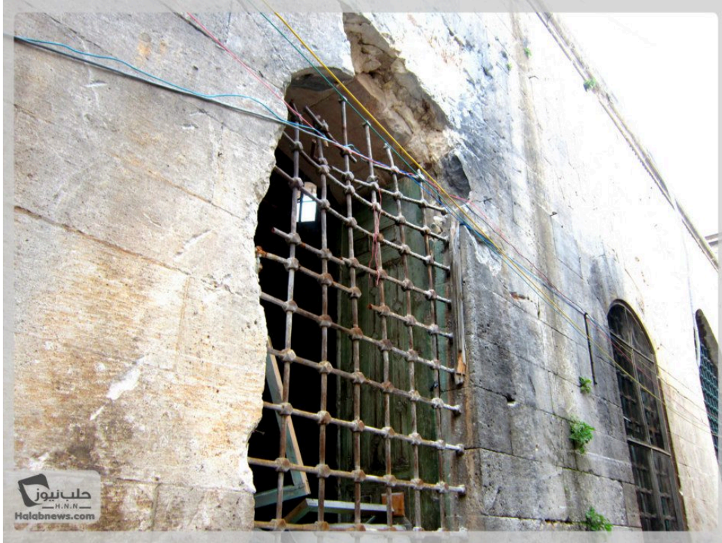
Combat damage sustained to the Madrasa al-'Utmaniya in Aleppo (APSA).
