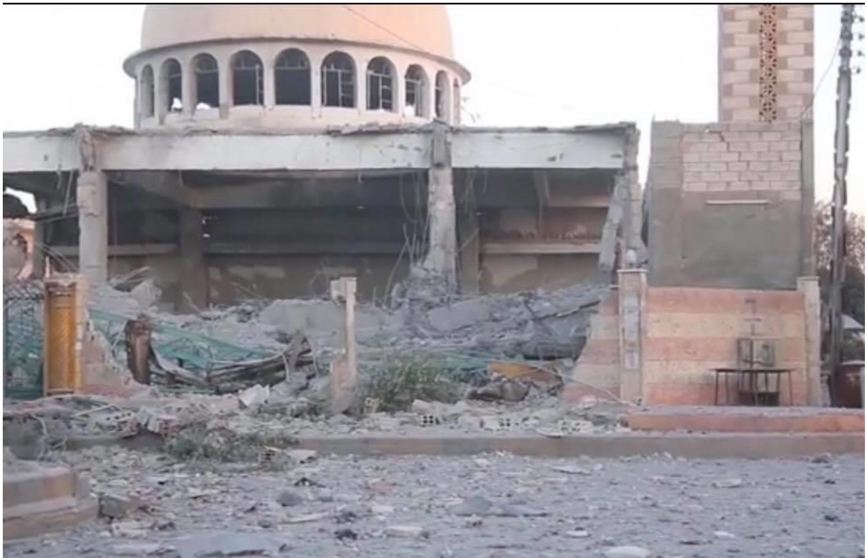
Damage to al-Nur Mosque (RBSS: June 10, 2017)
