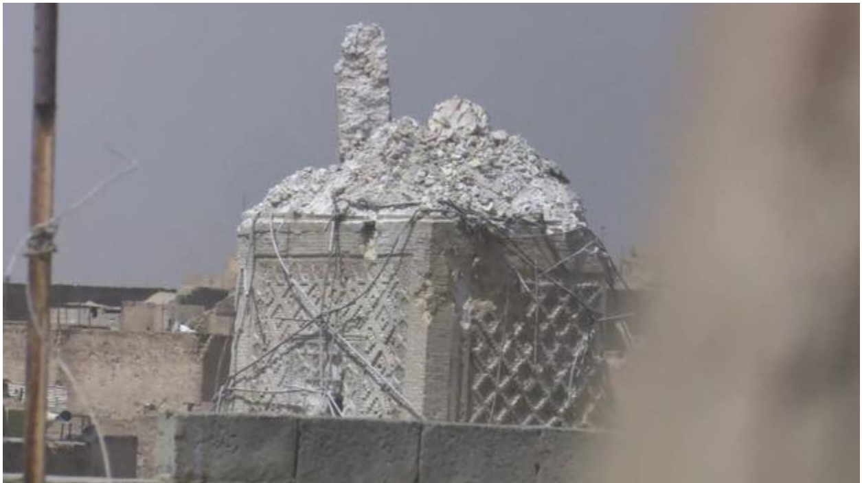
Detail of damage to al-Hadba Minaret (BBC; June 22, 2017)
