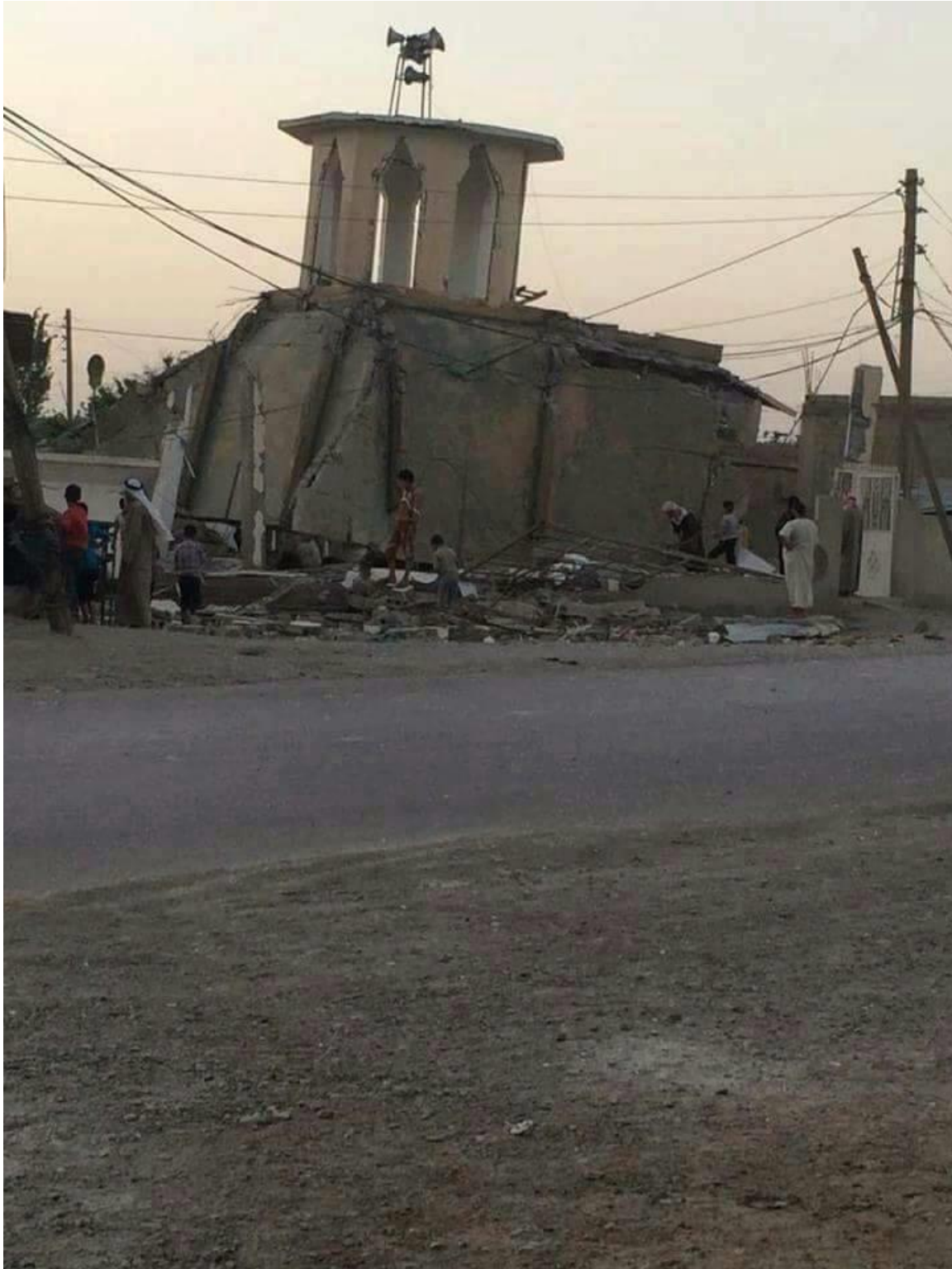
Damage to Abu Bakr al-Siddiq Mosque (SNHR; June 10, 2017)
