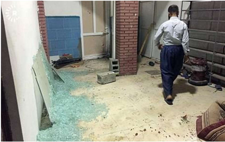
Damage to the interior of the mosque (Rudaw; June 16, 2017)
