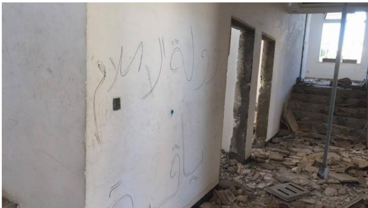
Graffiti on the walls of the basement and rubble on the floor (Fox News; June 14, 2017)
