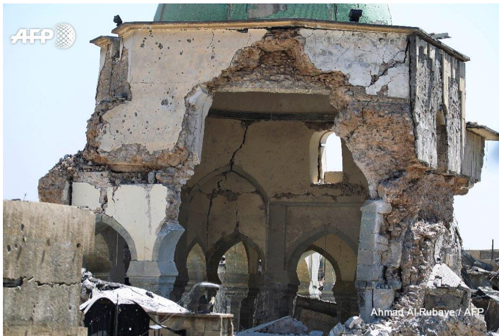
Detail of damage to al-Nuri al-Kabir Mosque (Ahmed Mousa; June 29, 2017)
