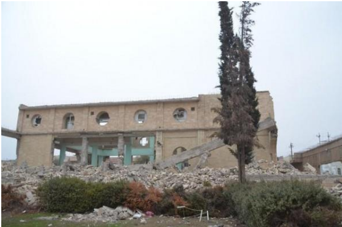
Damage to the exterior of the church (Ishtar TV; January 19, 2017)
