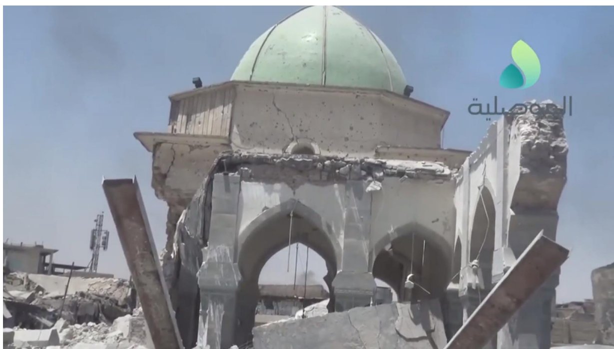
Damage to dome of al-Nuri al-Kabir Mosque (Al Mosuliya; June 30, 2017)
