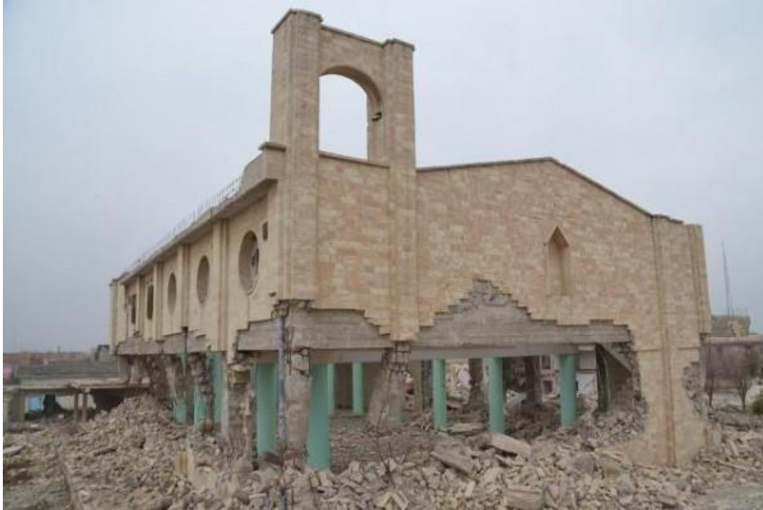
Damage to outside of church showing most of the walls of the first floor missing (Ishtar TV; January 19, 2017)
