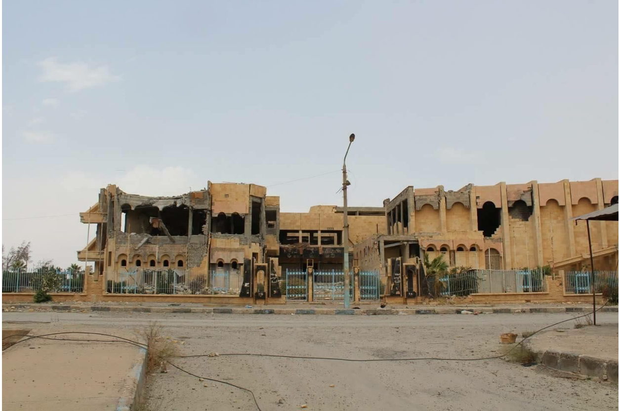
Tabqah Cultural Center with heavy damage to multiple parts of the building (RBSS; June 7, 2017)
