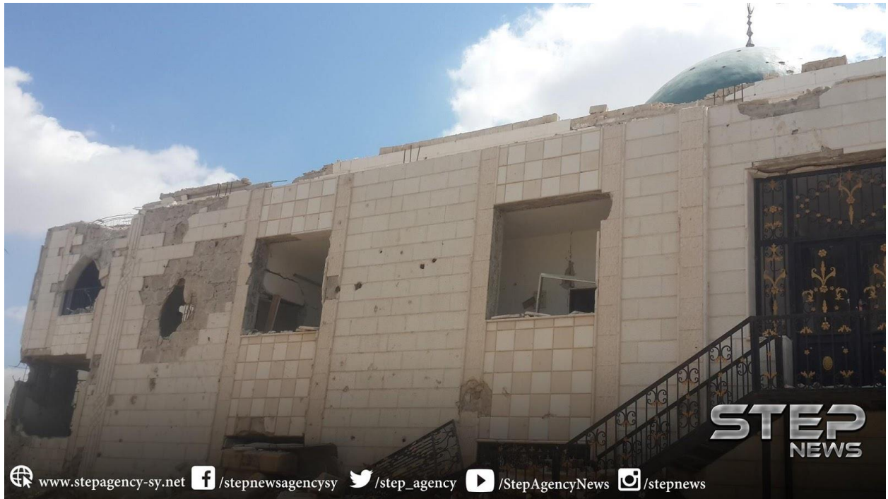
Damage to al-Rahman Mosque, seen from the west (Step News Agency; June 20, 2017)
