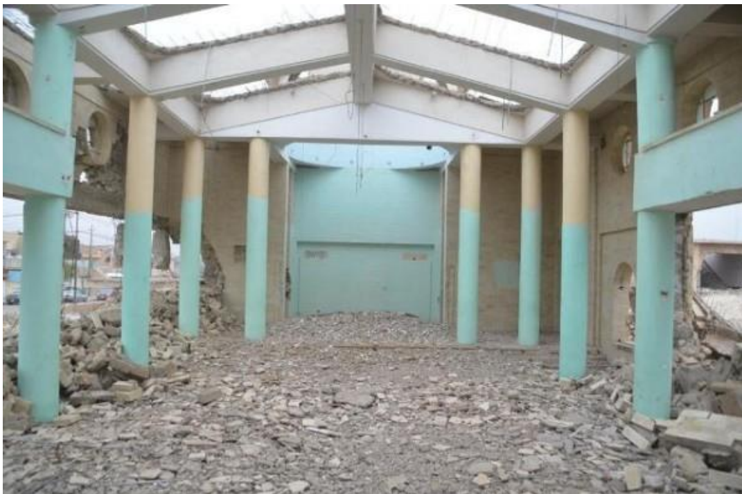
Damage to the interior of the church, looking towards where the altar was located (Ishtar TV; January 19, 2017)
