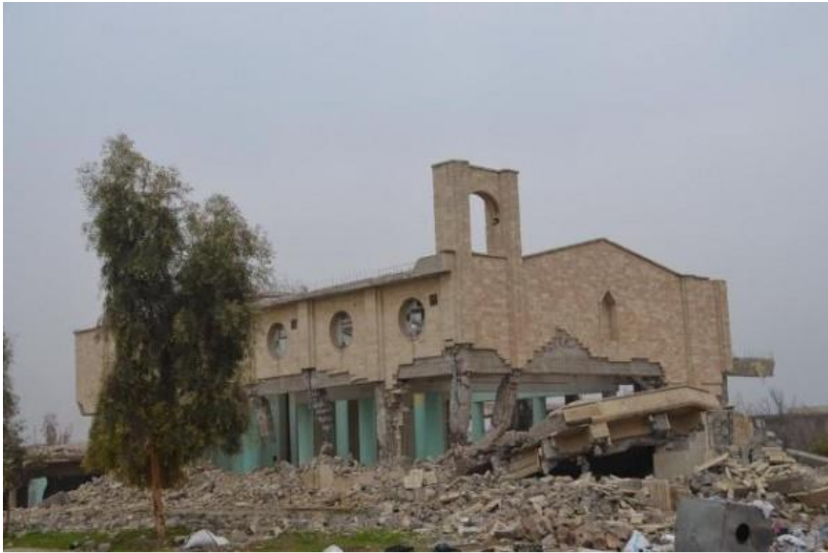
Damage to the outside of the church (Ishtar TV; January 29, 2017)
