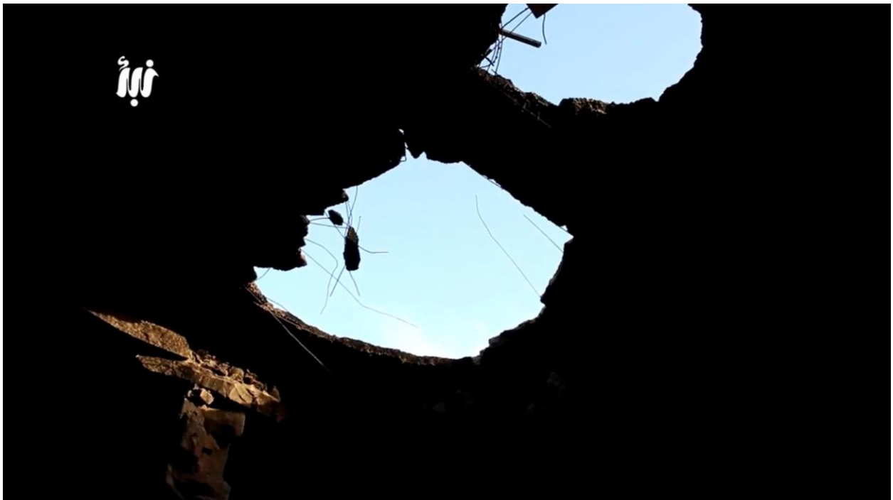
Video still of damage to the roof of the portico (Nabaa; June 9, 2017)
