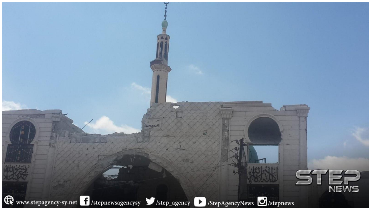
Damage to al-Rahman Mosque, seen from the north (Step News Agency; June 20, 2017)
