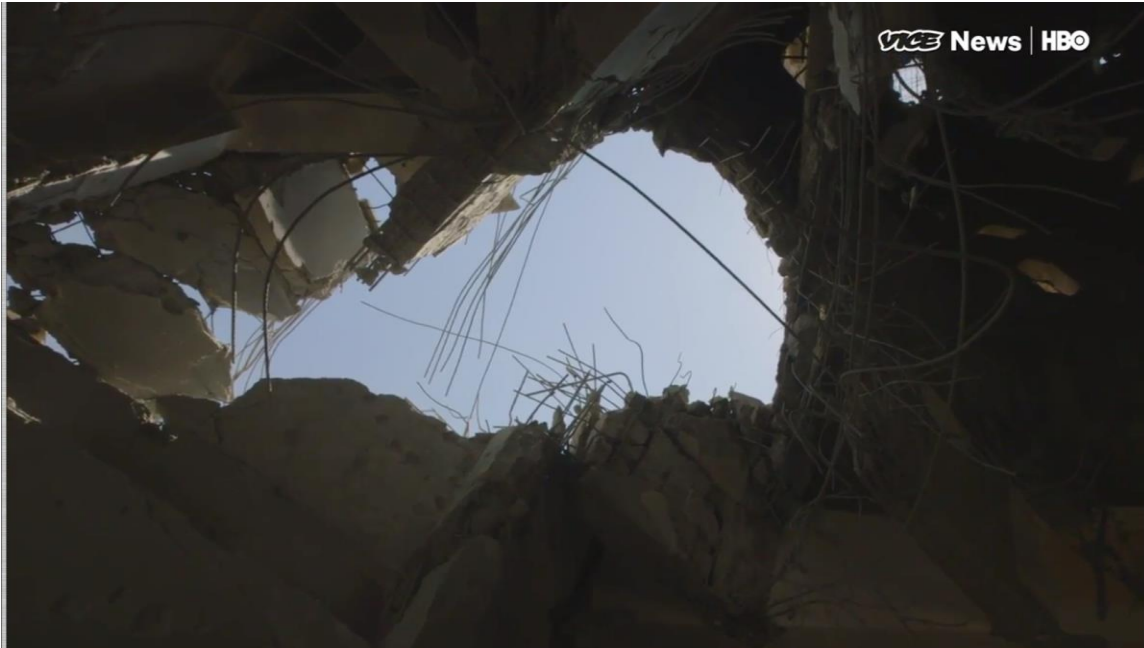
Damage to interior of al-Imam Muhsin Mosque (Vice News; June 30, 2017)
