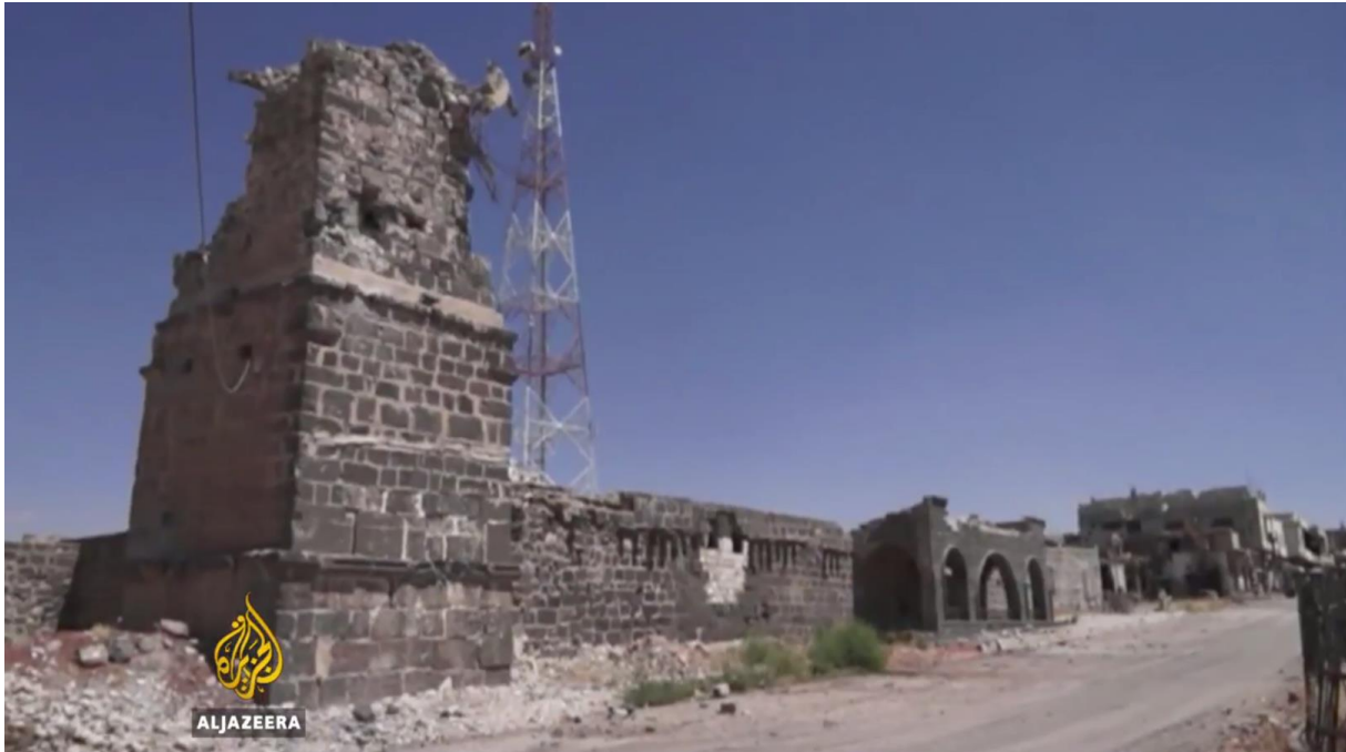
Damage to mosque and minaret (Al Jazeera; June 26, 2017)
