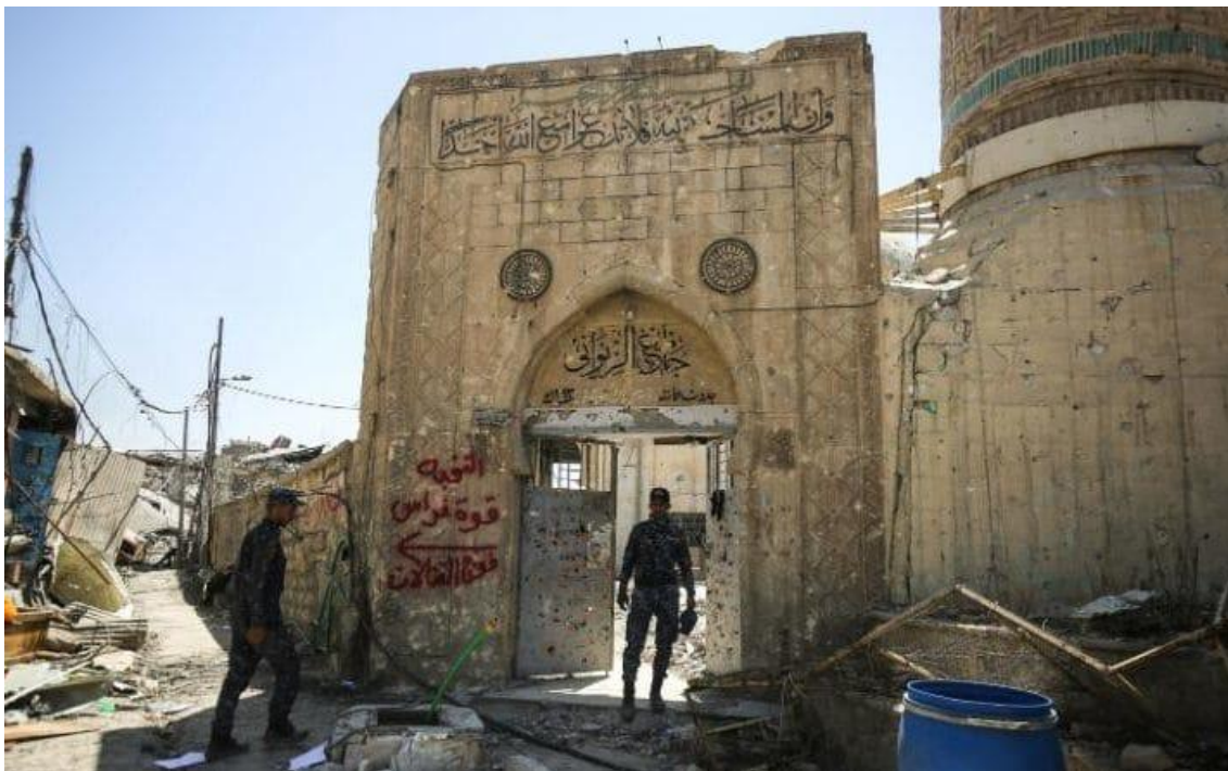
Damage to al-Zewani Mosque (Telegraph; June 29, 2017).
