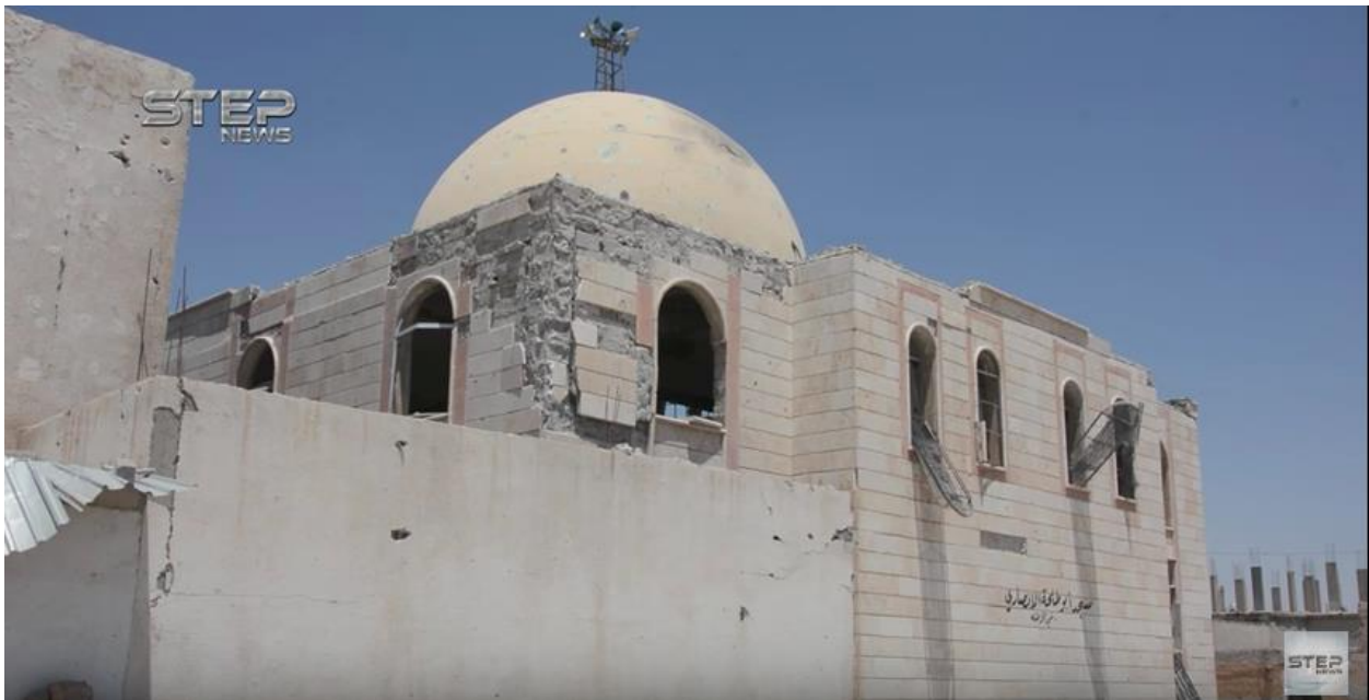
Video still showing damage to al-Subaiha Mosque (Step News Agency; June 12, 2017)
