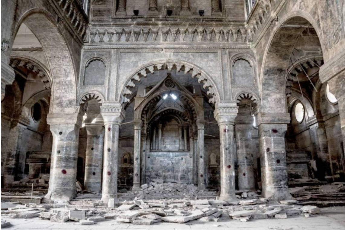
The interior of Mar Thomas showing damaged altar, ceiling pieces on the floor, and black dots painted on columns (L'Orient Le Jour/Elizabeth Fitt; July 1, 2017)
