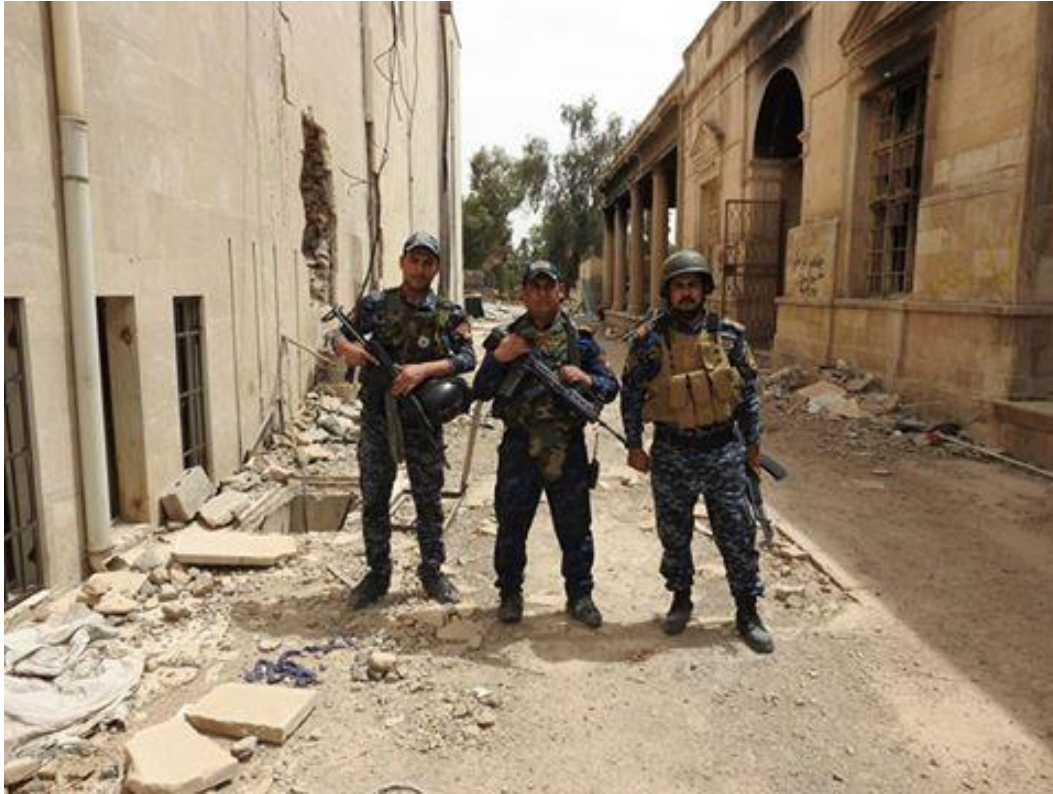
Damage to the side of the Mosul Museum, the large hole visible in the wall is due to previous damage (Personal Facebook Account; June 15, 2017)
