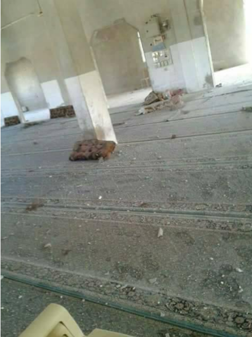
Damage to the interior of Abu Bakr al-Sadeiq Mosque (SNHR; June 2, 2017)
