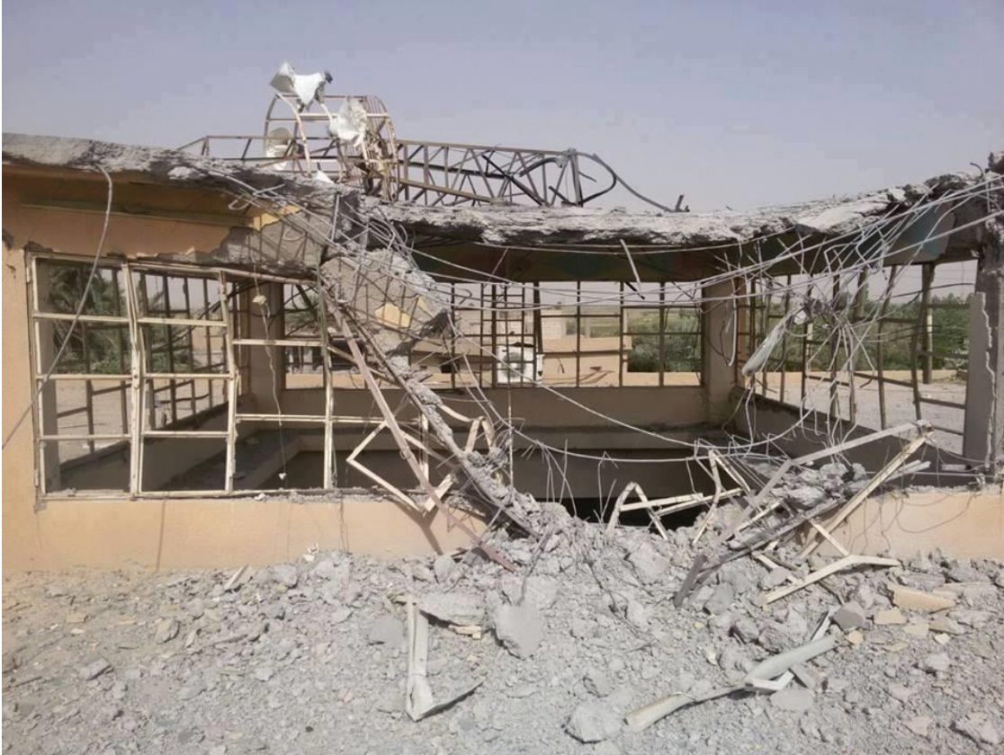
Damage to the roof of Abu Bakr al-Sadeiq Mosque (SNHR; June 2, 2017)
