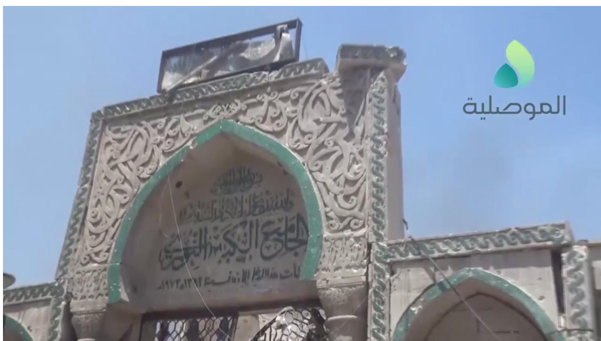
Detail of damage to main gate of complex (Al Mosuliya; June 30, 2017)
