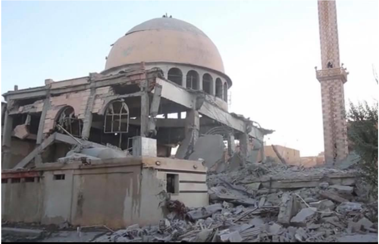
Damage to al-Nur Mosque (RBSS: June 10, 2017)
