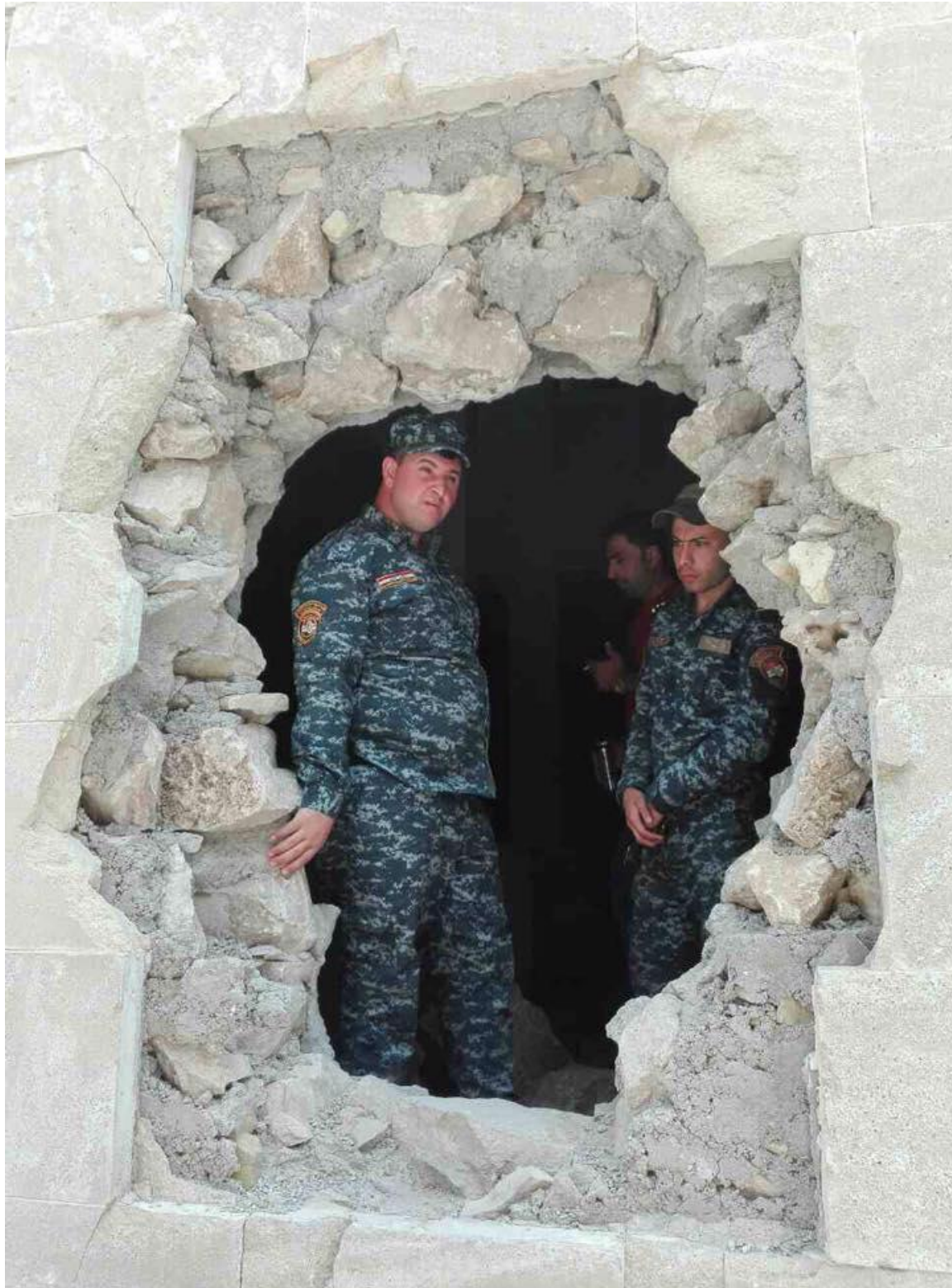
Detail of large hole in side of Mosul Museum (Personal Facebook Account; June 14, 2017)
